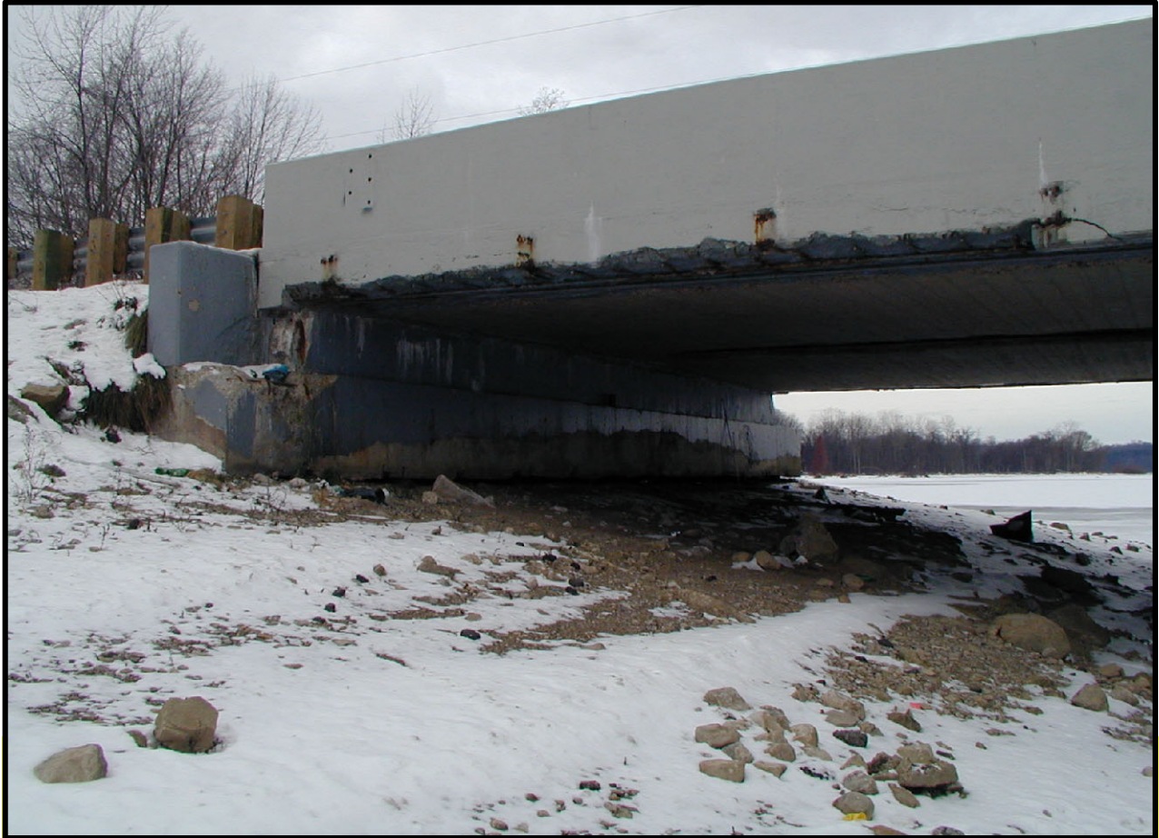
▲ Photo #1. Facing southwest. Note the undermining of the start (south) abutment. ULTV is (3 LF, 44 LF, 7 inches).
