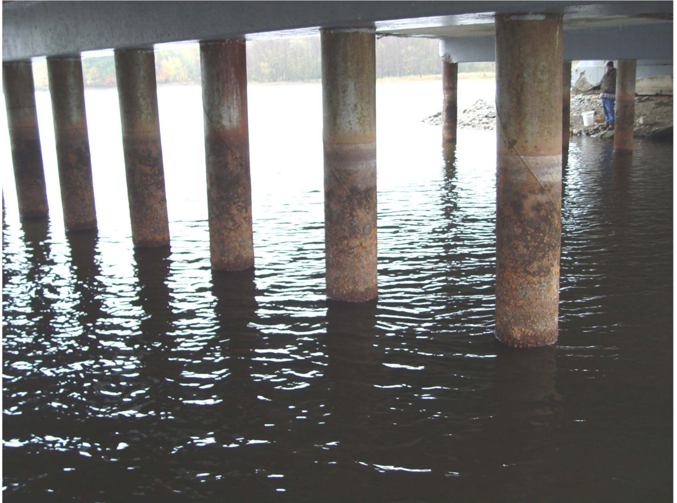
Photo 2. Facing north looking at the steel pile columns of Pier 1. Note the rusting section loss occurring at the waterline.
