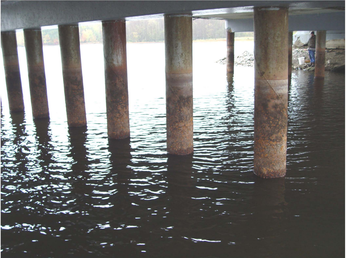
Photo 2. Facing north looking at the steel pile columns of Pier 1. Note the rusting section loss occurring at the waterline.
