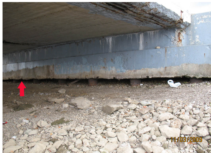
P6: START (S) ABUTMENT. NOTE PILE EXPOSURE. ARROW IS NEAR CENTERLINE OF BRIDGE.
