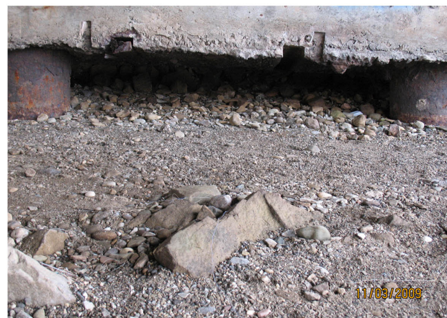
P7: CLOSE-UP OF ARROW IN P6. EROSION IS STARTING TO GET BEHIND ABUTMENT.
