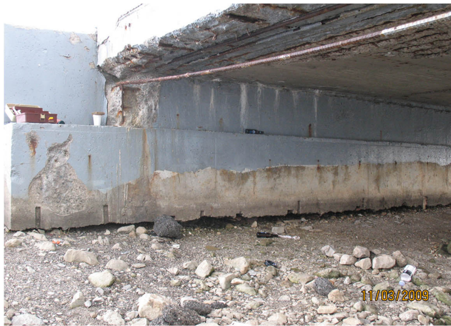
P4: FINISH (N) ABUTMENT. NOTE MOST OF DECK EDGE SPALLS ARE UNDER OLD RAILING. NEW RAIL WAS ADDED TO THE INSIDE OF OLD.
