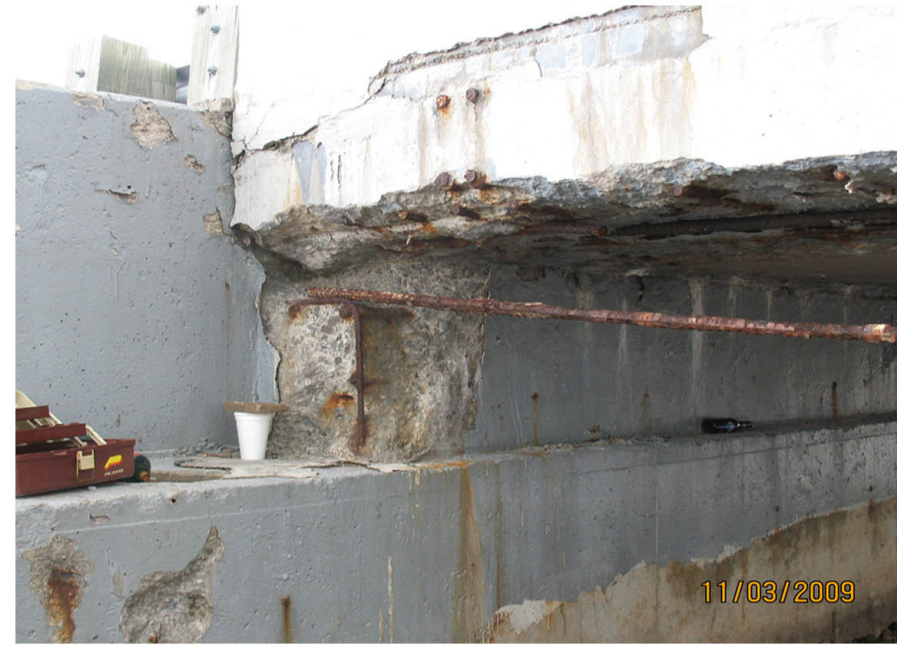
P5: DETERIORATED FINISH-LEFT (NW) ABUTMENT. NOTE REBAR HANGING WAS REMOVED ON 11/6/09.
