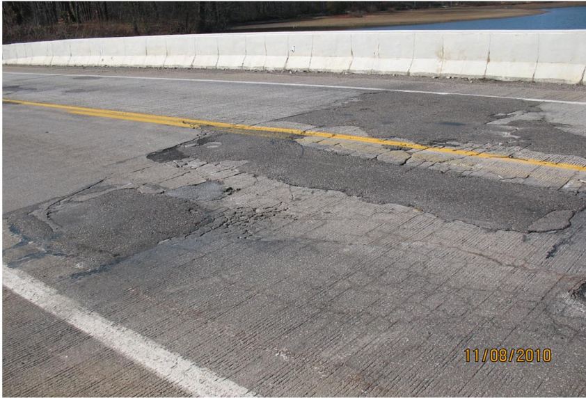
P5: LARGE ASPHALT PATCHES AND BREAKING UP AREAS OVER MID-SPAN.
