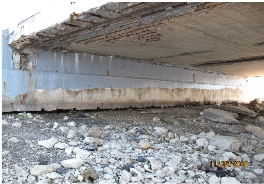
P9: FORWARD ABUTMENT UNDERMINED.
