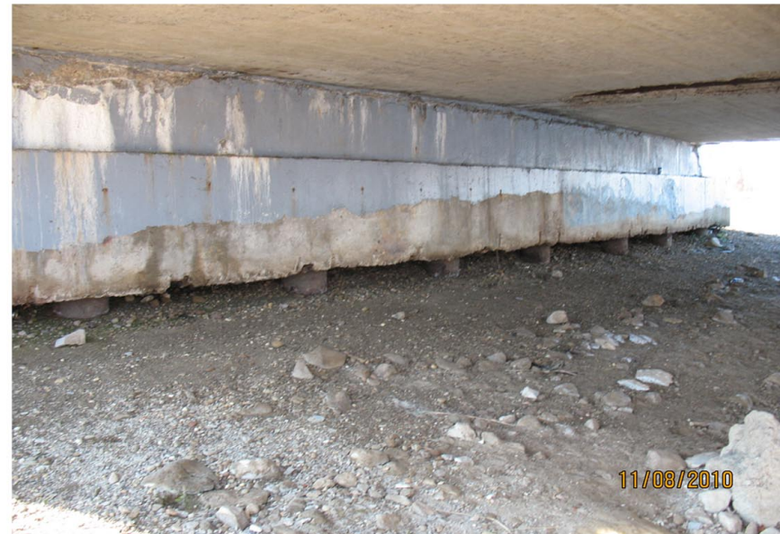
P12: REAR ABUTMENT UNDERMINED. A FEW AREAS OF THE UNDERMINING ARE STARTING TO GET BEHIND BACKWALL HERE.
