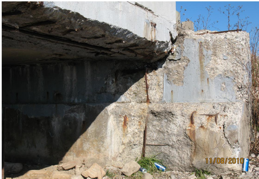
P11: FORWARD ABUTMENT SEAT LOSS UNDER NORTHEAST CORNER OF THE DECK.
