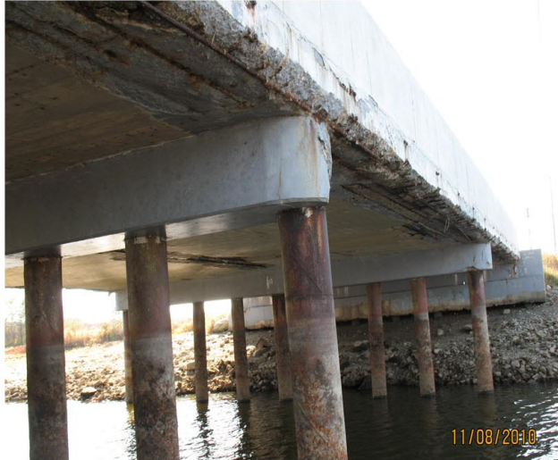
P5: TYPICAL EDGE SPALLING.
