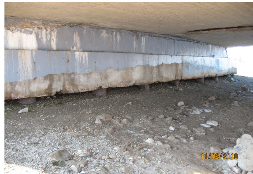
P12: REAR ABUTMENT UNDERMINED. A FEW AREAS OF THE UNDERMINING ARE STARTING TO GET BEHIND BACKWALL HERE.
