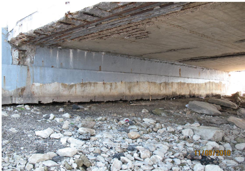
P9: FORWARD ABUTMENT UNDERMINED.
