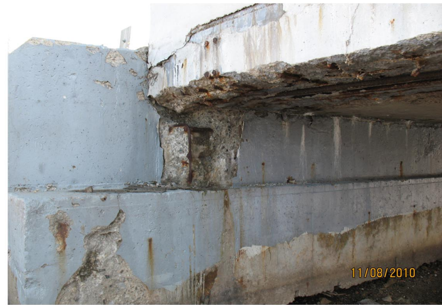
P10: FORWARD ABUTMENT SEAT LOSS UNDER NORTHWEST CORNER OF THE DECK.
