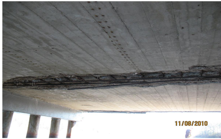
P2: LOOKING EAST IN SPAN #1. NOTE 360 DEGREE REBAR EXPOSURE
