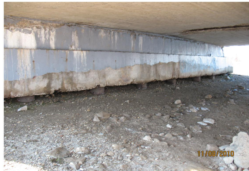
P12: REAR ABUTMENT UNDERMINED. A FEW AREAS OF THE UNDERMINING ARE STARTING TO GET BEHIND BACKWALL HERE.
