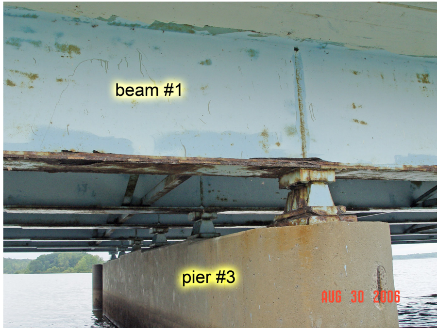
P1 rusting section loss of beam #1 at pier #3.psd
