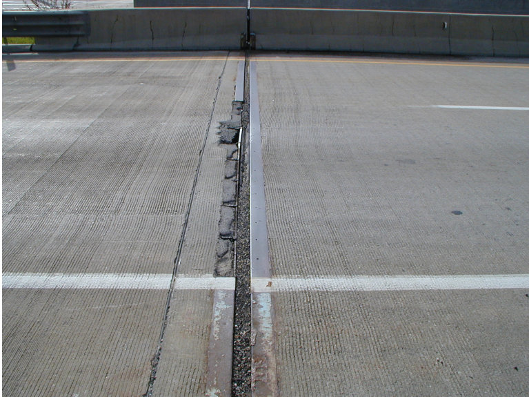
PHOTO #1 12 FOOT OF THE APPROACH SLAB SIDE OF THE DECK ARMOR, WAS CUT OUT IN LANE #2.
