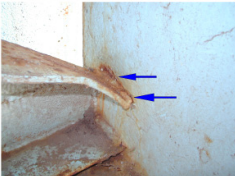
PHOTO #4 ARROWS SHOW A 1-1/2" CRACK OF THE EAST ABUTMENT END FRAME ANGLE WELD TO THE INSIDE BEAM WEB OF THE SOUTH FASCIA.
