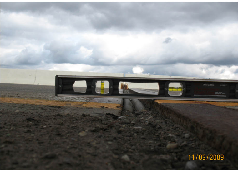
P6: BRIDGE DECK IS A 1/2" LOWER THEN APPROACH SLAB. MEASUREMENT IS TAKEN BY ARROW IN P1 ABOVE.
