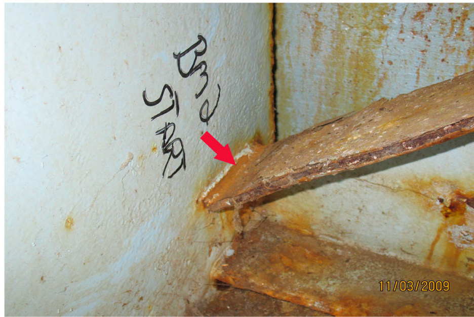
P7: ARROW SHOWS CRAKED ENDFRAME WELD TO BEAM #2 AT START (E) ABUTMENT.
