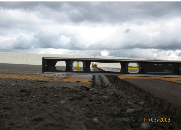
P6: BRIDGE DECK IS A 1/2" LOWER THEN APPROACH SLAB. MEASUREMENT IS TAKEN BY ARROW IN P1 ABOVE.
