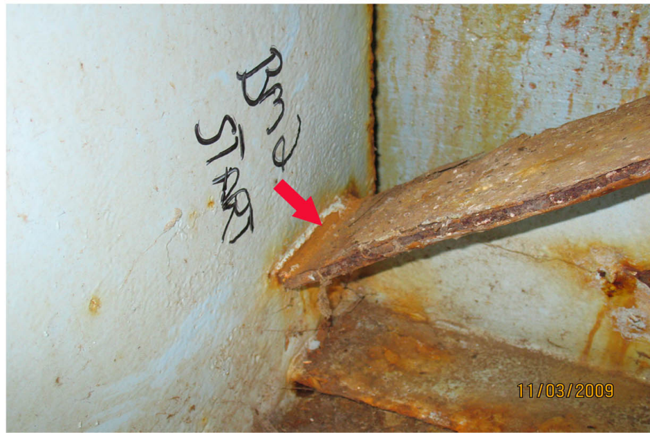
P7: ARROW SHOWS CRAKED ENDFRAME WELD TO BEAM #2 AT START (E) ABUTMENT.
