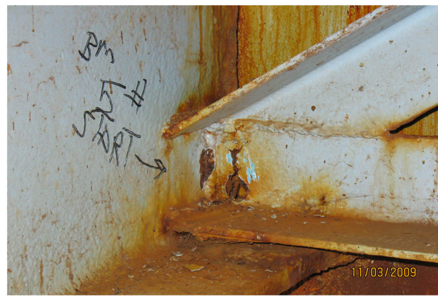
P7: CRACKED AND RUSTING THRU HOLE TO START (W) ENDFRAME AT BEAM #5.
