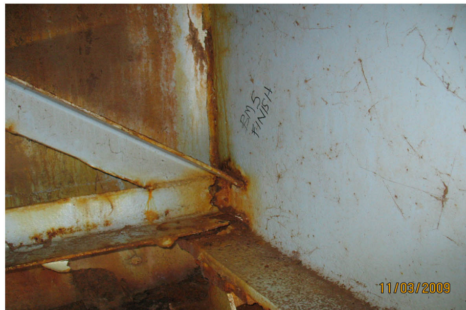
P8: SEVERED ENDFRAME AT FINISH ABUTMENT TO BEAM #5.
