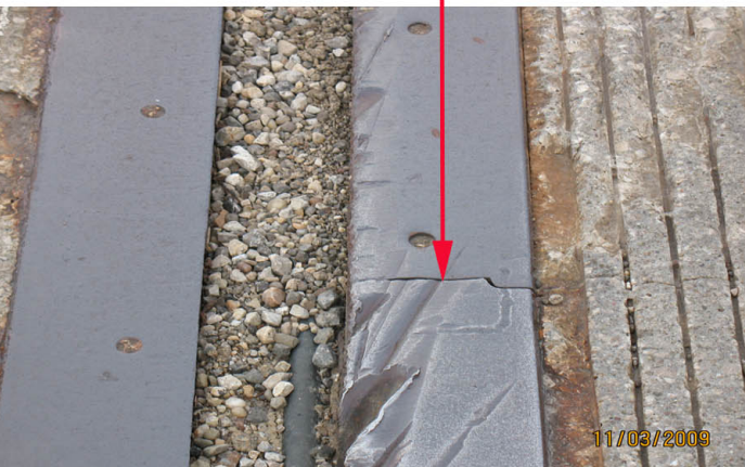
P1 - P4: SHOWS EAST EXJT. NOTE MANY GOUGES, MISSING AND CRACKED ARMOR. MOST DAMAGE IS TO LANE #2 EASTBOUND.
