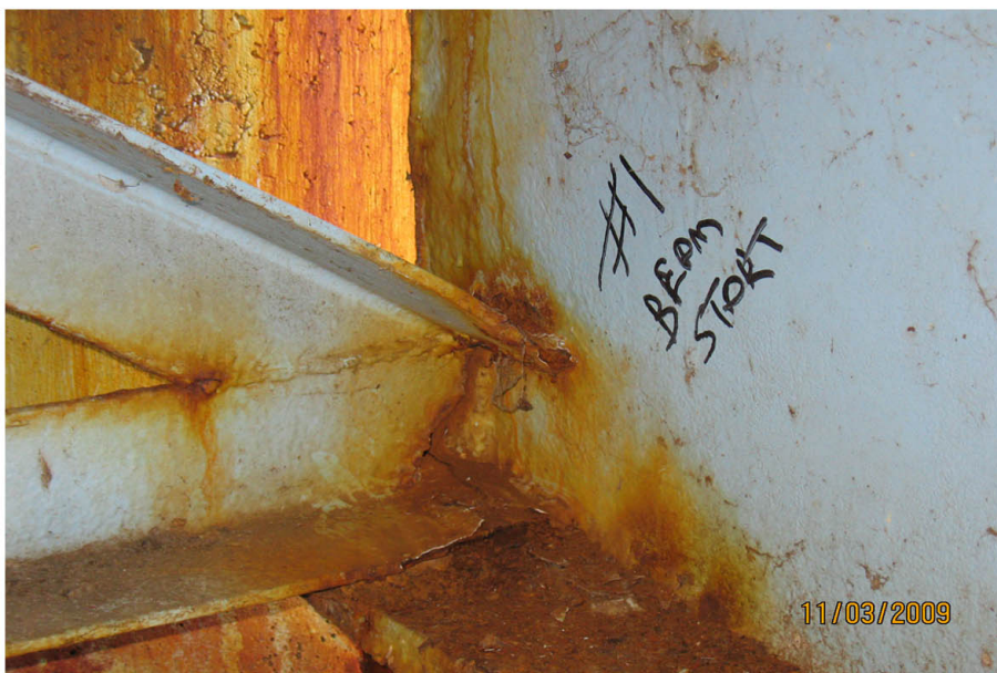
P6: START (W) ABUTMENT AT BEAM #1. CRACKED ENDFRAME. WEB OF BEAM HERE FLEX'S WITH HEAVY LOAD.
