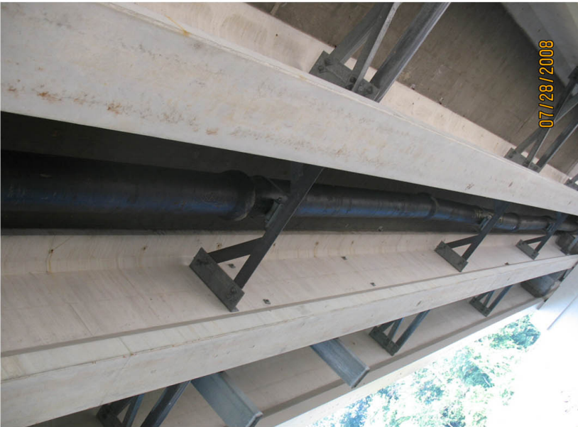
P3: TYPICAL MISALIGNMENT OF 16" PIPE IN BAY #3
