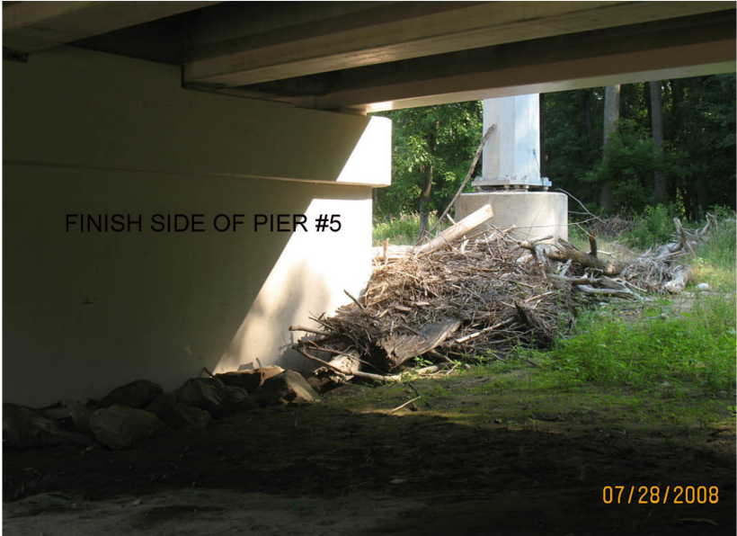
P4: NOTE LOG JAM BETWEEN PIER 5 AND UTIL POLE FOUNDATION. HIGH WATER FLOWS THRU HERE.
