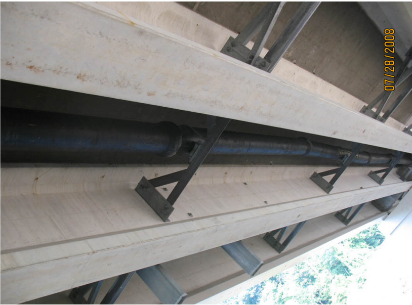
P3: TYPICAL MISALIGNMENT OF 16" PIPE IN BAY #3
