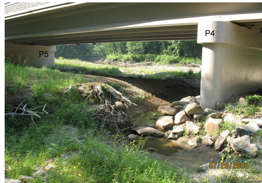
P6: THIS IS THE PATH OF THE RED LINE IN P5. NOTE SOME WASH OUT TO FINISH SIDE OF PIER #4.
