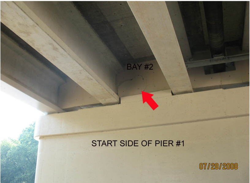
P1: 5 SF DELAM TO CONCRETE DIAPHRAGM.
