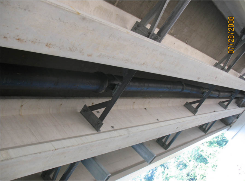
P3: TYPICAL MISALIGNMENT OF 16" PIPE IN BAY #3
