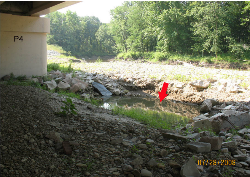
P7: THIS IS THE PATH OF THE BLUE LINE IN P5. NOTE THE SMALL POND THAT THE ARROW IS POINTING TO. POND IS AS DEEP AS 3 FT.
