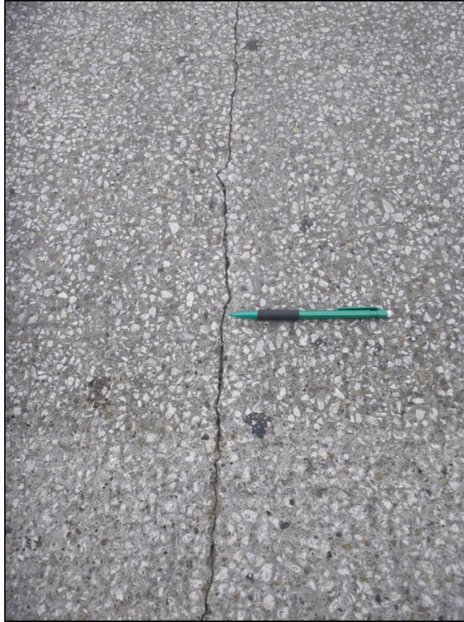
Picture #11: Full width 1/8" crack in eastbound wearing surface near Sta. 990+60, looking north.
