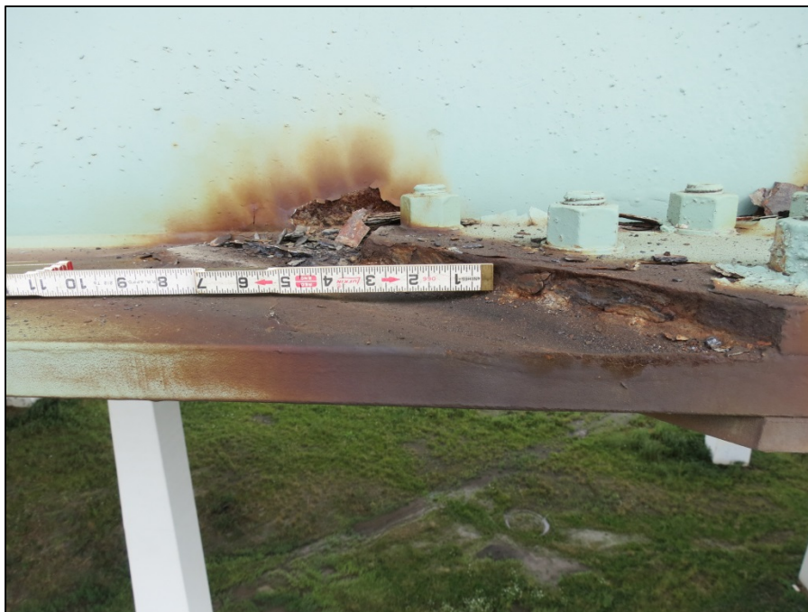
Picture #27: 1/4" section loss to exterior half of girder M bottom flange in span 8R, looking north.
