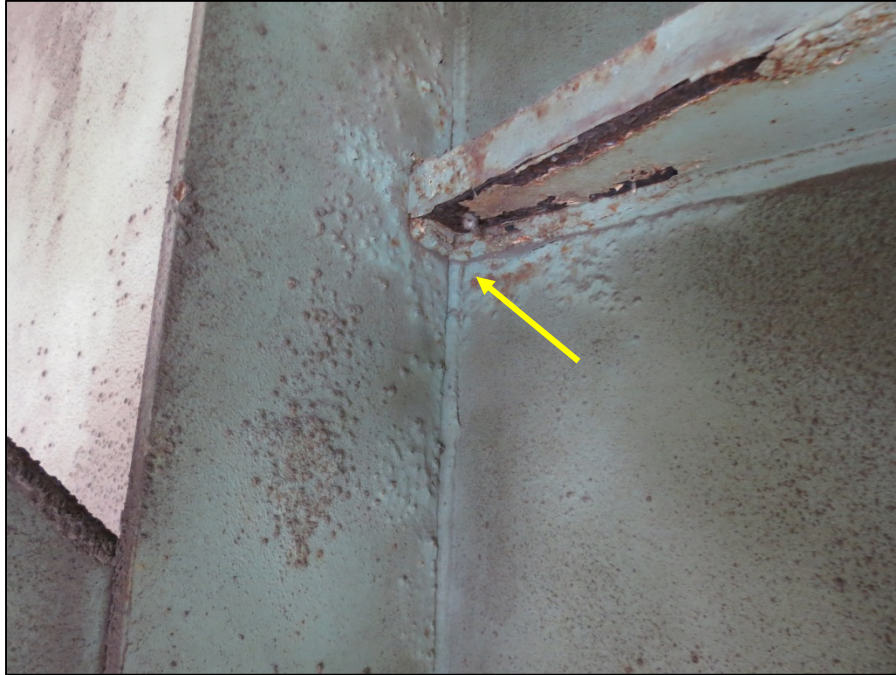
Picture #43: Tri-axial weld on girder V, span 21R, looking north.
