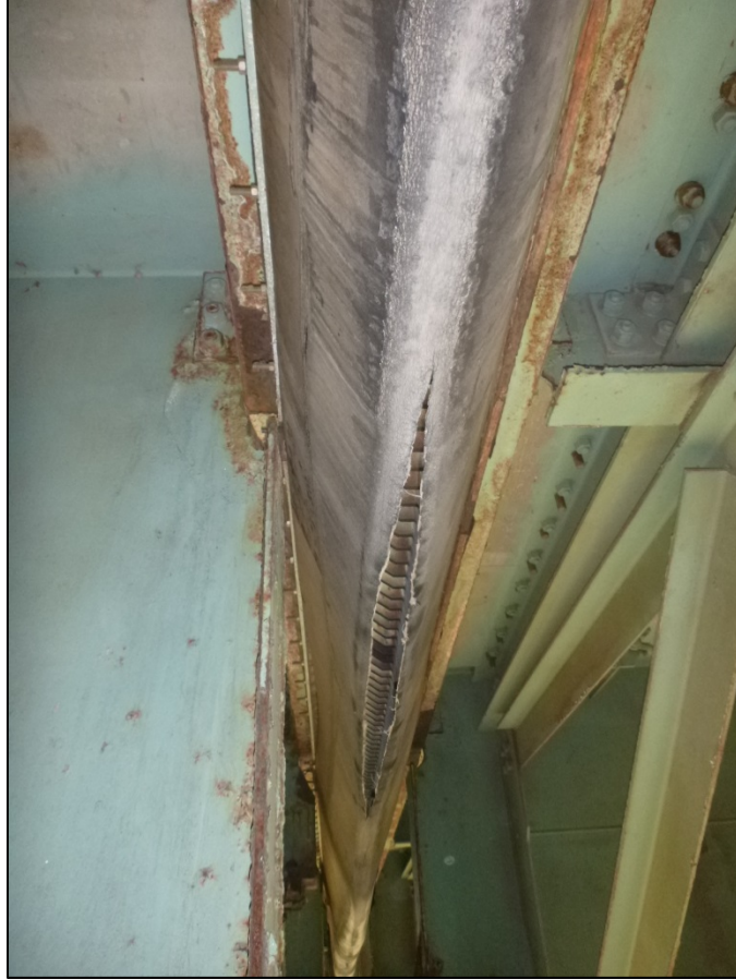
Picture #19: Failed neoprene trough at roller 4R, girder G, looking south.
