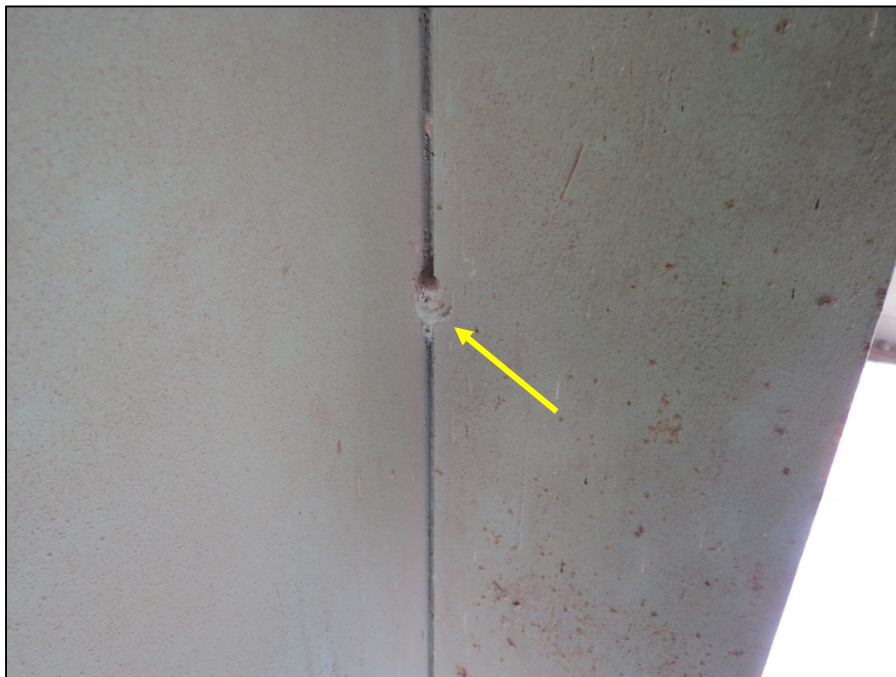
Picture #44: Tack weld on web of girder J in span 14R, looking north.
