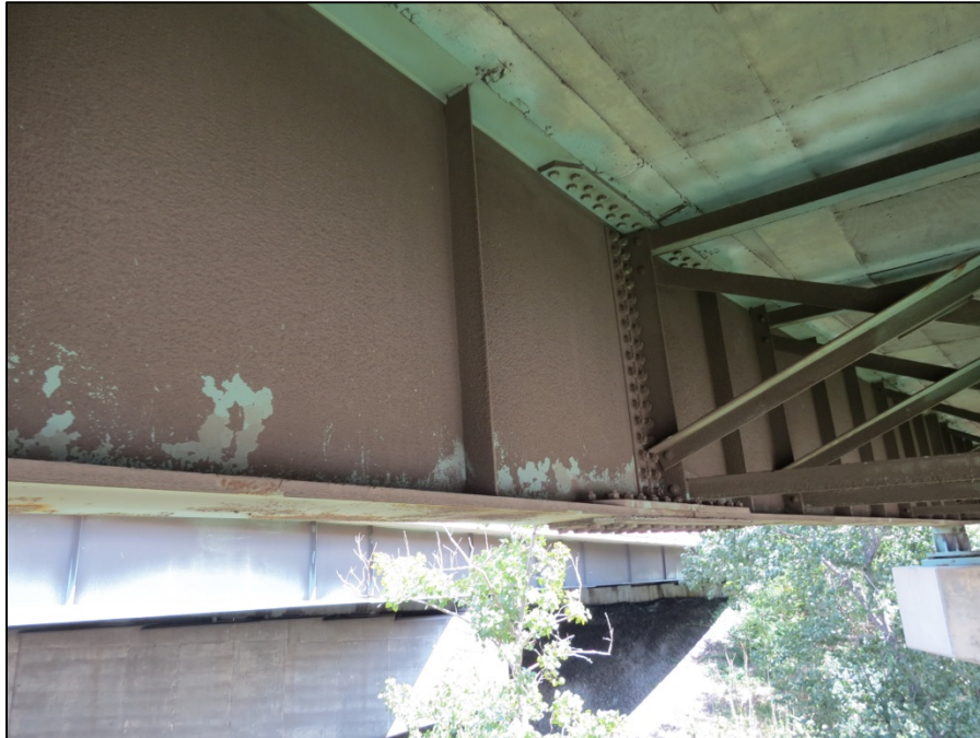
Picture #41: Dirt build up on web of girder CB-A in span 24CB, looking east.
