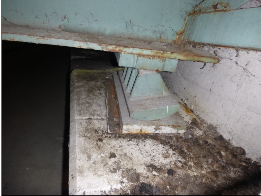
Picture #39: West abutment bearing 1-EA leaning 17° east at 75°F, looking south.
