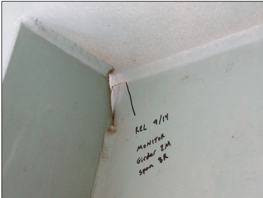
Picture #29: Possible 1" crack near girder M compression flange in span 8R, looking south.
