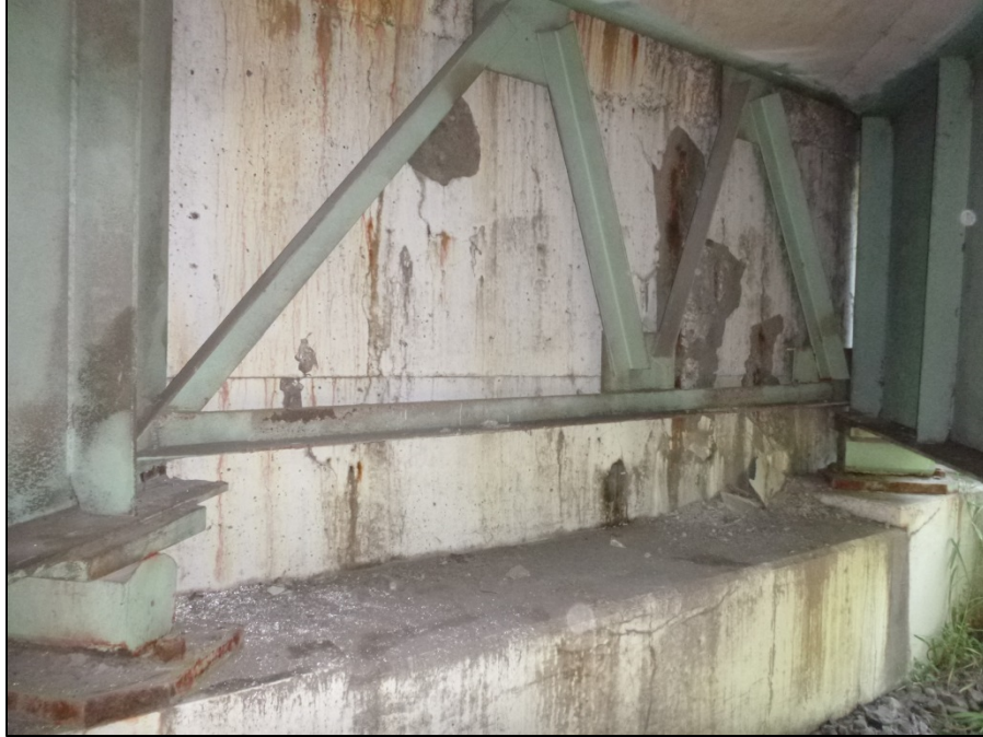
Picture #48: Large spalls and delamination on ramp C-B abutment backwall between girders D and E, looking east.
