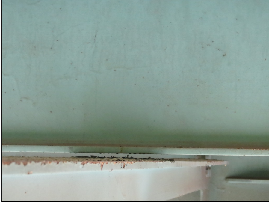
Picture #34: 3/4" gap between stringer 5 and floorbeam 6 in span 7L, looking north.
