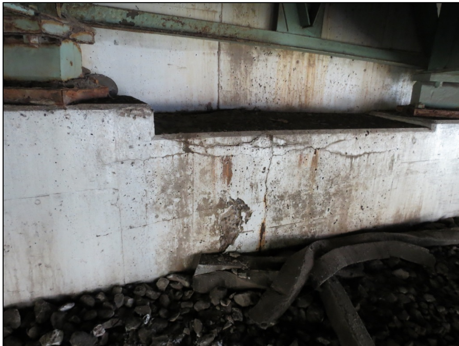
Picture #45: Deterioration to forward abutment wall between girders E and F, looking east.
