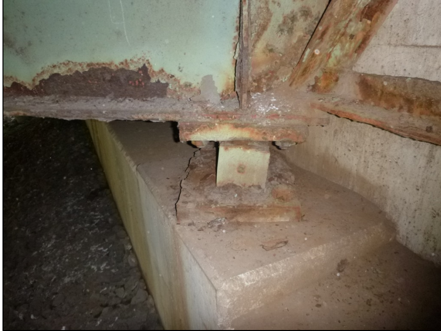
Picture #37: Rust and debris around girder 6-G rocker at forward abutment, looking north.
