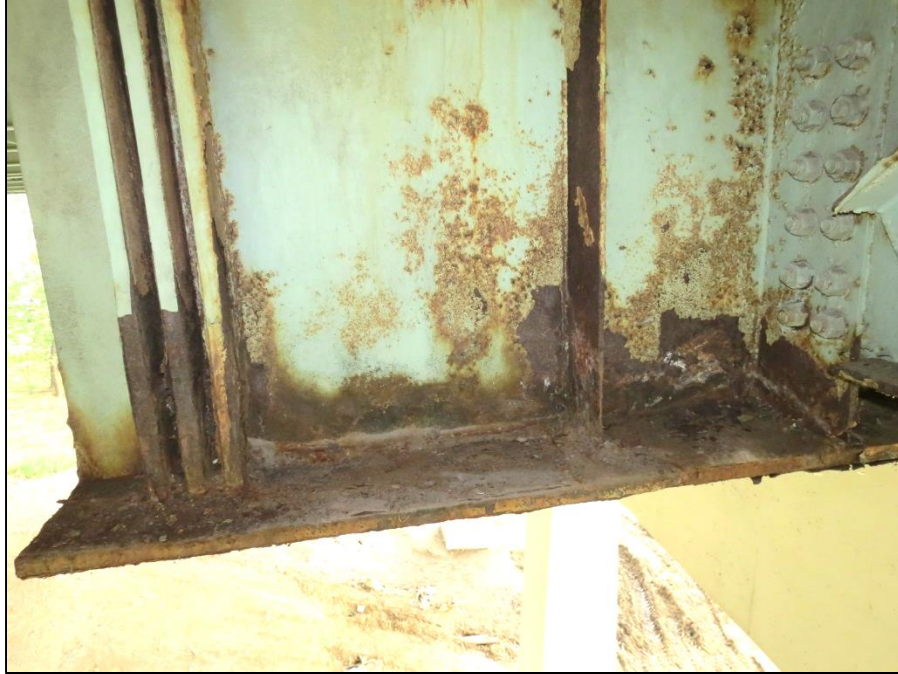
Picture #28: Section loss to girder F bottom flange in span 4L, looking north. Note bottom of transverse stiffener is nearly rusted through.
