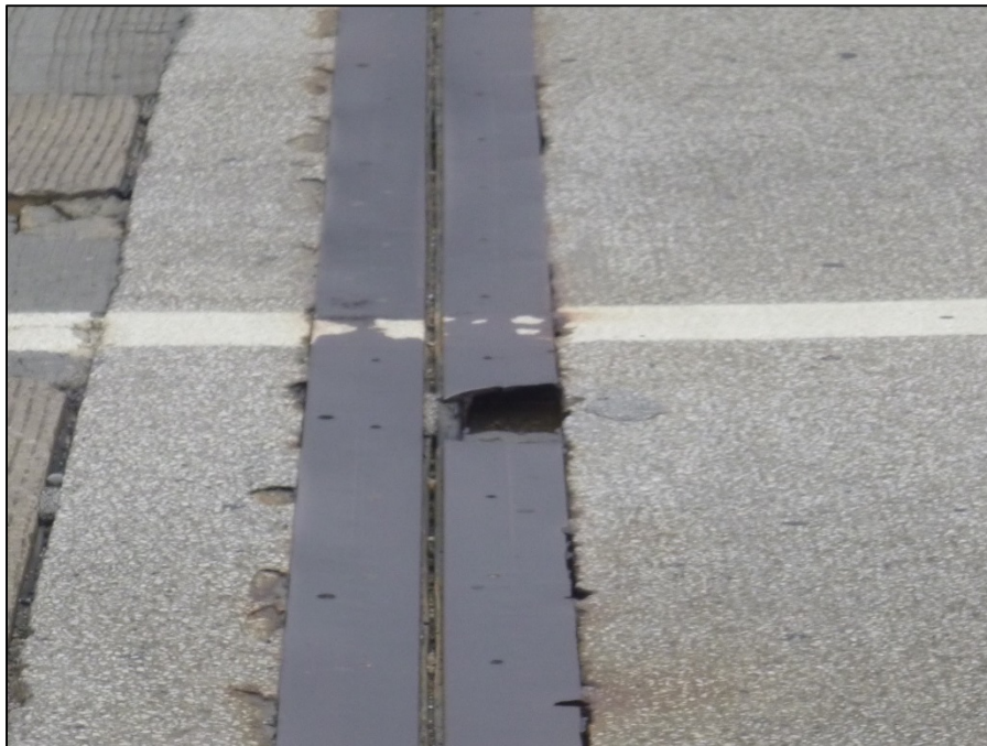
Picture #23: Deep hole below broken joint armor near lane 3/4 lane line at eastbound rear abutment, looking north.
