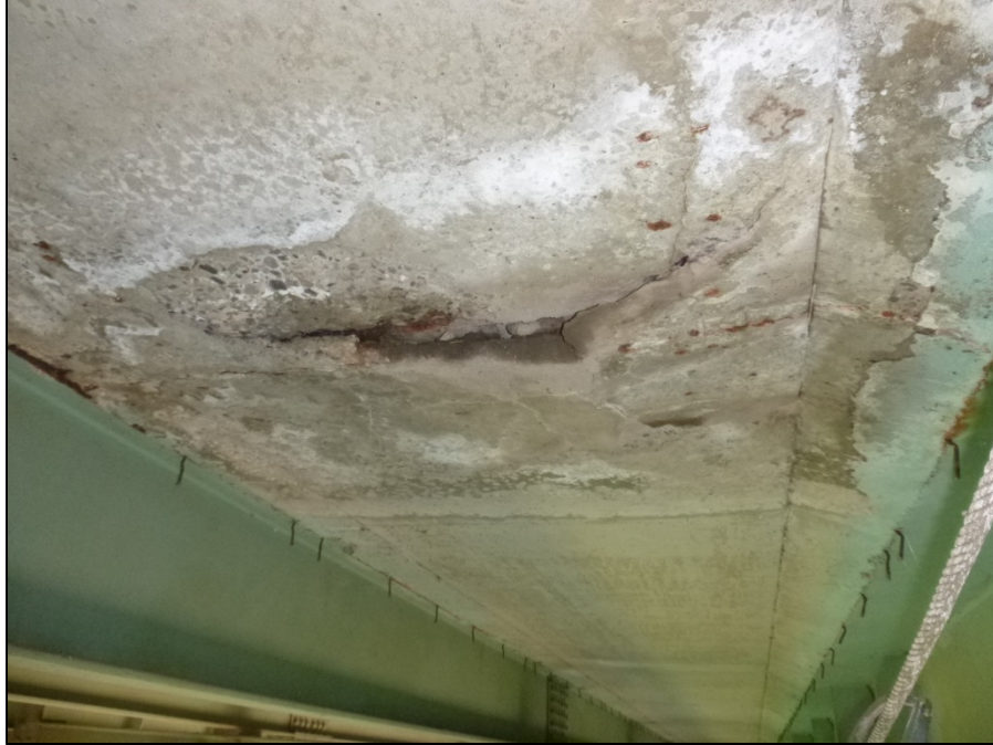
Picture #6: Spalled and delaminated underside of deck between girder 4-B and stringer 4-3 in span 14L over Independence Road.
