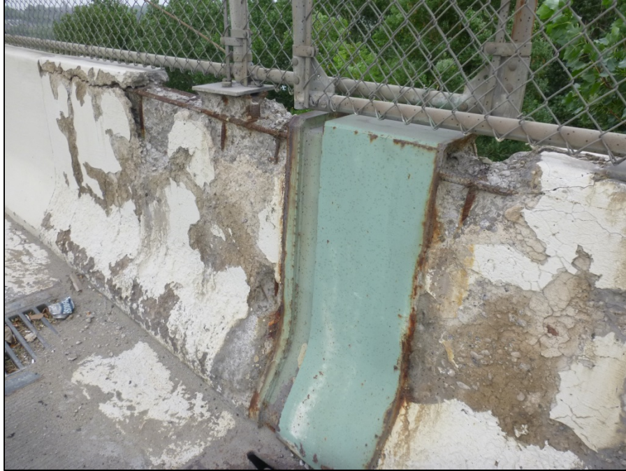
Picture #15: Cracked, spalled, and scaled concrete on westbound railing at expansion joint 4, looking north.
