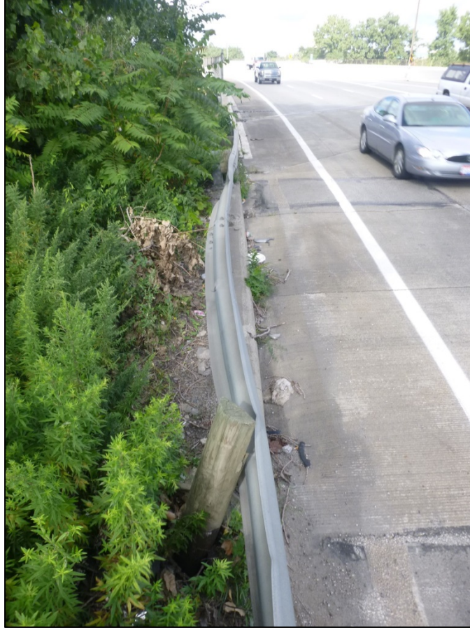
Picture #4: Three consecutive posts sheared off or missing at the eastbound forward approach, looking west.
