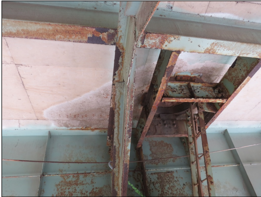
Picture #8: Typical deck saturation around pier access manhole. Eastbound deck over pier 14R shown, looking south.
