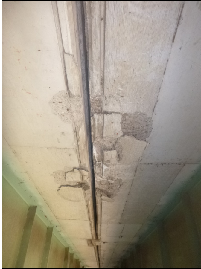
Picture #9: Multiple spalls in span 19 with exposed reinforcing steel, looking east.
