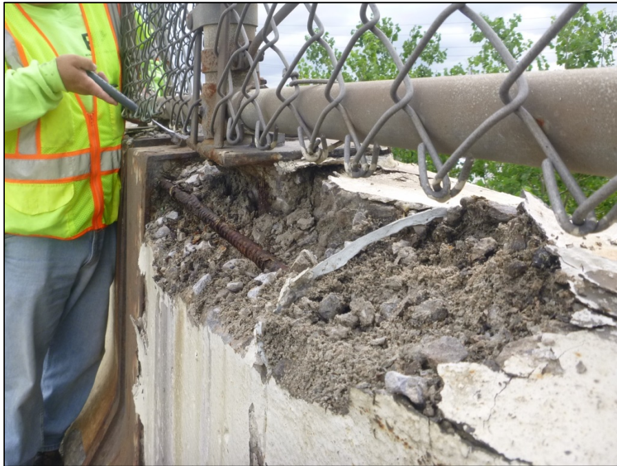
Picture #14: Concrete deterioration on eastbound railing at expansion joint 1, looking east. Note the fence post is now unsupported.
