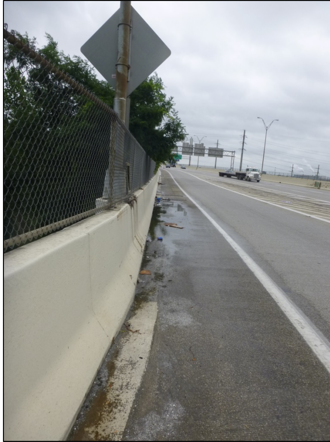
Picture #17: Ponding adjacent to two scuppers on westbound deck in Unit 1, looking east. Note the trees overhanging the fence onto the deck.
