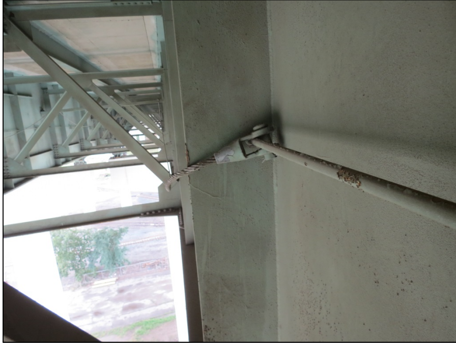
Picture #52: Safety cable improperly attached to handrail on south face of girder D at floorbeam 7, span 11L, looking west.
