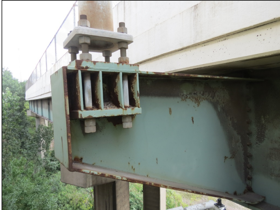
Picture #50: Eastbound exit sign support in fair condition with debris and minor section loss, span 23R, looking east.
