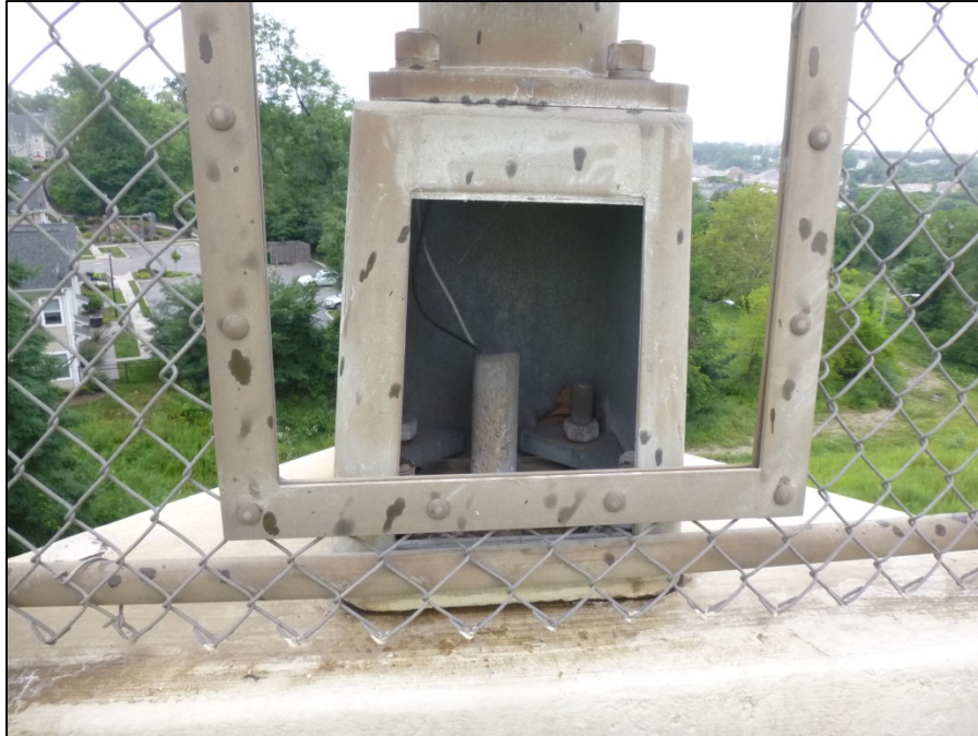
Picture #51: Missing electrical cover plate exposing westbound light pole wiring at Sta. 991+35, looking north.
