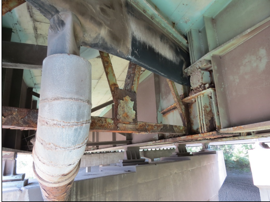
Picture #31: South bay hinge crossframe in span 24 C-B, looking west. Up to 50% section loss on members.
