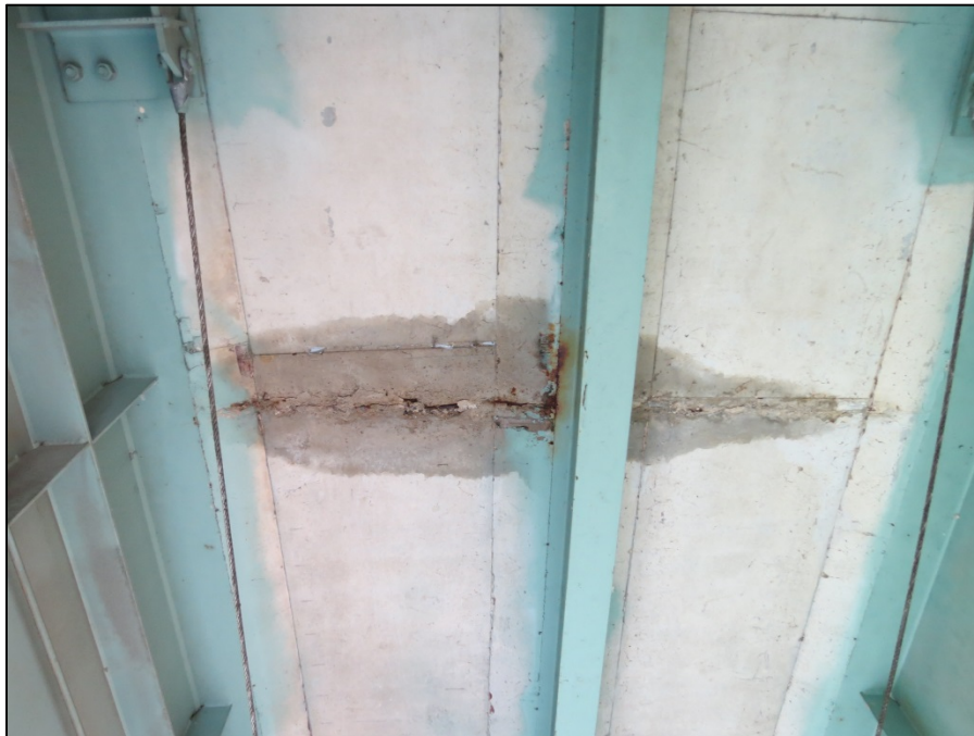
Picture #5: Typical leaking deck construction joint in span 6L between girders A and C, looking east. Note minor deterioration to stringer top flange.
