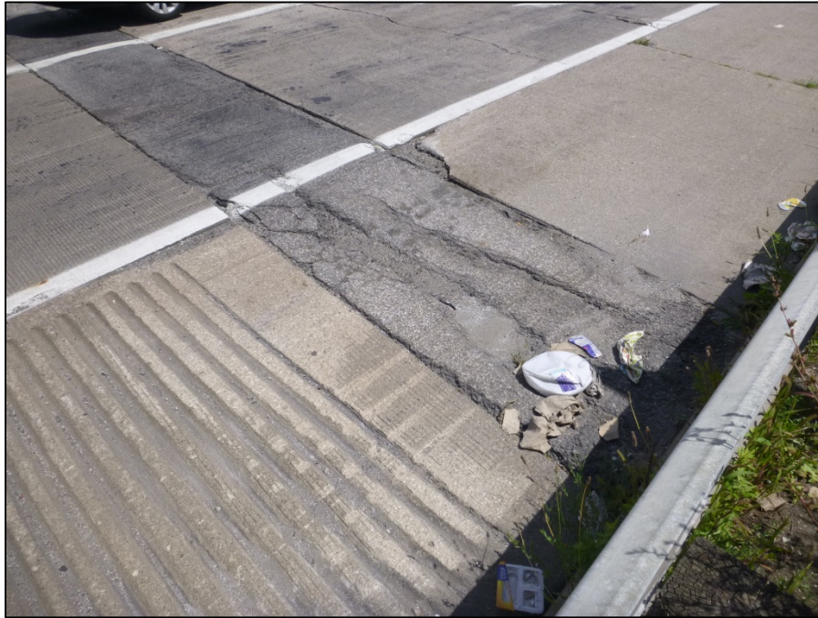
Picture #3: Cracking asphalt in the south shoulder and settled pavement in the lanes at the pavement relief joint at eastbound Ramp C-B to Broadway Avenue.
