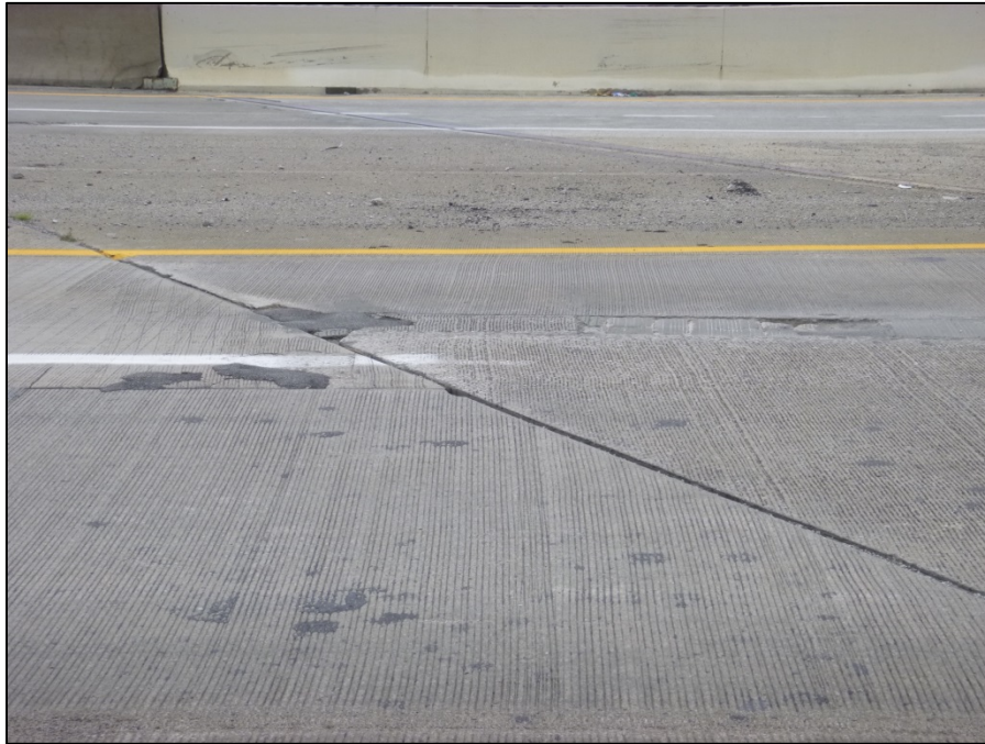
Picture #2: Westbound forward approach slab patches deteriorating, looking south.
