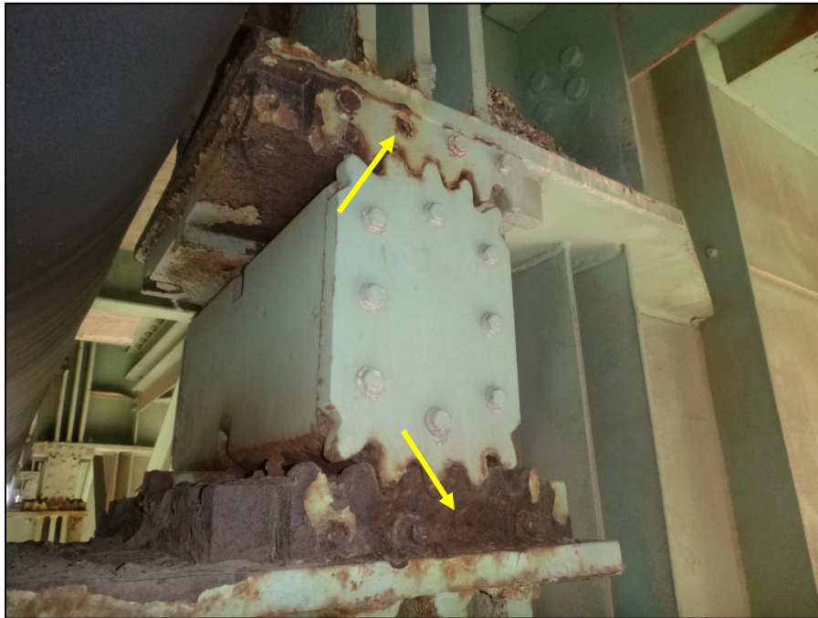
Picture #42: Broken/missing bolts on girder D roller 3 alignment plate, looking north.
