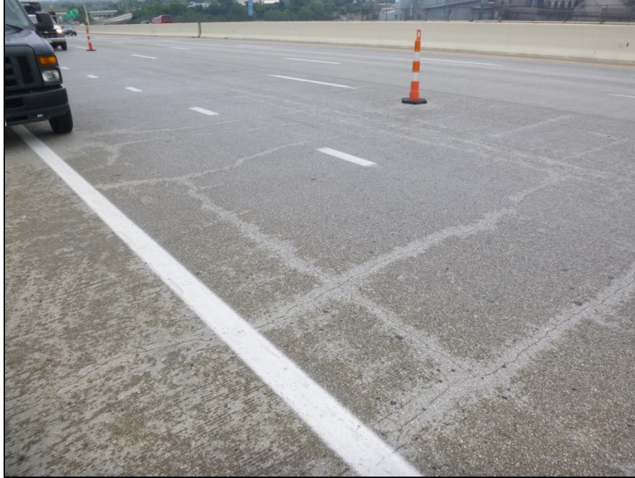
Picture #10: Typical cracking in wearing surface, unit 4, westbound deck, looking south.
