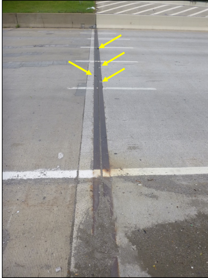
Picture #22: Multiple holes in the eastbound rear abutment steel joint armor , looking north.
