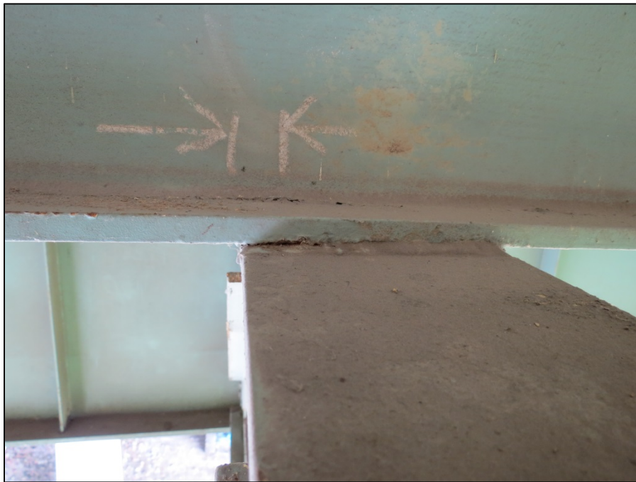
Picture #33: 1.75” crack in stringer 13 to floorbeam 3 weld in span 5R, looking north.
