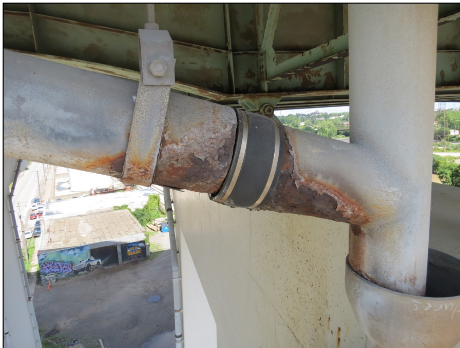
Picture #18: Downspout coupler separated near pier 9R, girder 3-K, looking north.
