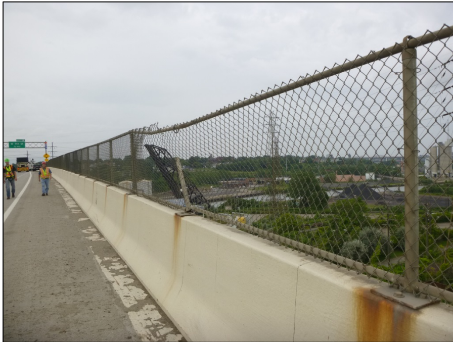
Picture #16: 20 feet of damaged westbound fence, including broken post, in Unit 4 at Sta. 1007+88, looking northwest.
