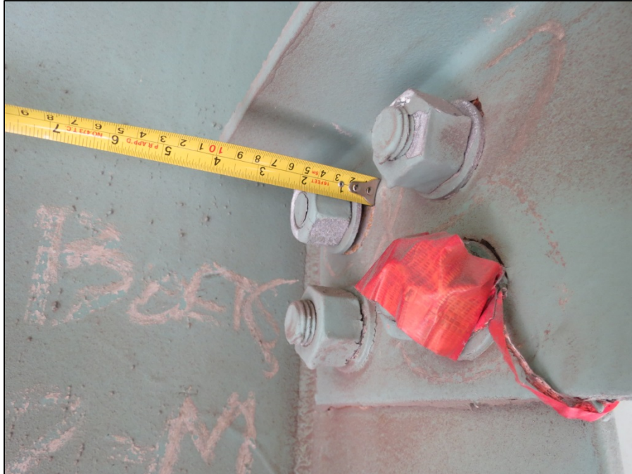
Picture #35: All 4 bolts in floorbeam top chord connection to girder M loose, span 9R, looking southwest.
