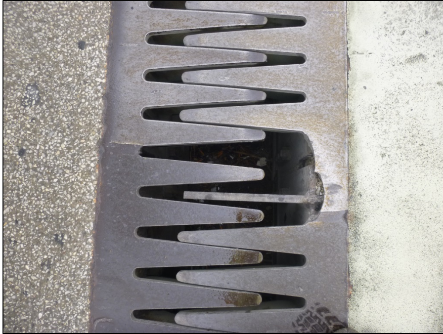
Picture #25: Missing finger in westbound intermediate expansion joint 2, lane 4, looking south.
