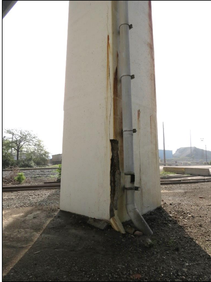
Picture #47: Large delaminations, spalls, and cracks with rust staining and efflorescence on south column of pier 9R, looking south.
