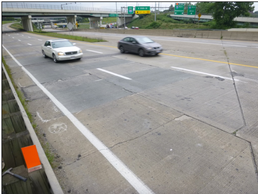
Picture #1: Westbound forward approach pavement exhibits cracks and asphalt patches.
