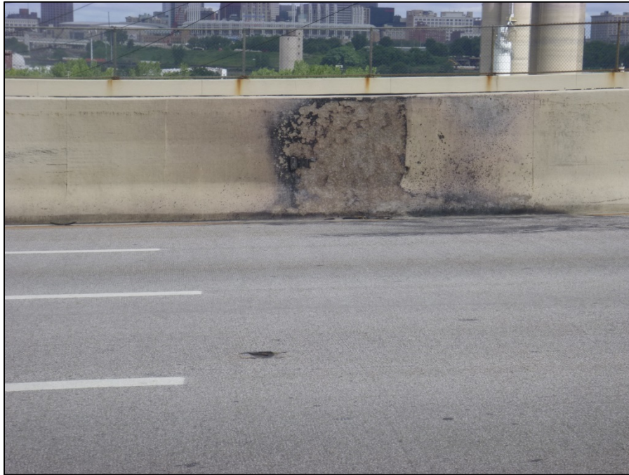
Picture #13: Fire damage to Unit 2 eastbound median barrier near Sta. 992+00, looking north.
