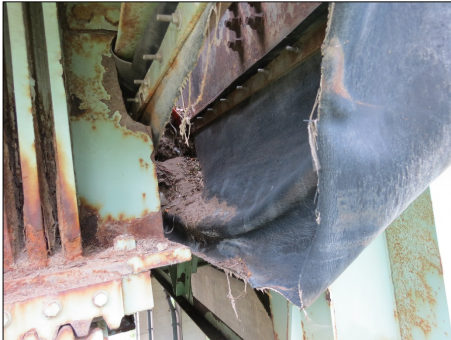
Picture #20: Failed neoprene drainage trough at roller 4L, girder A, looking south.
