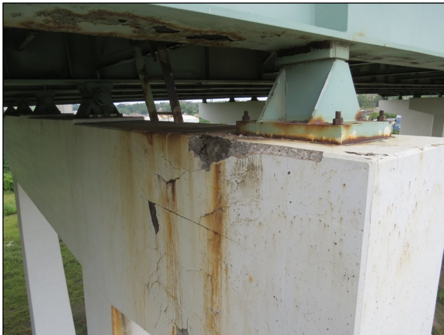
Picture #46: Deterioration to south end of pier 7R cap due to leaking deck access manhole, looking east.
