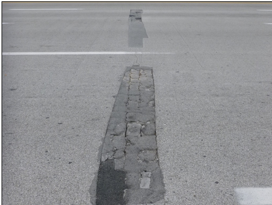
Picture #12: Deteriorating patch at full width transverse crack in westbound deck over pier 14, looking south.
