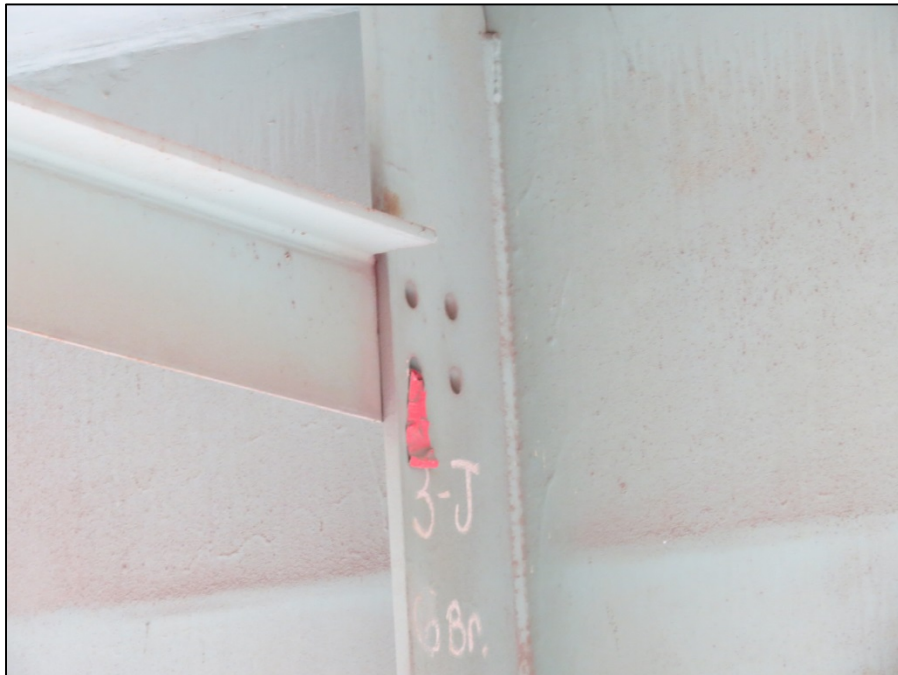
Picture #36: All 4 bolts in floorbeam top chord connection to girder J missing, span 11R, looking southeast. Note, this is the 1 foot of floorbeam rated critical.
