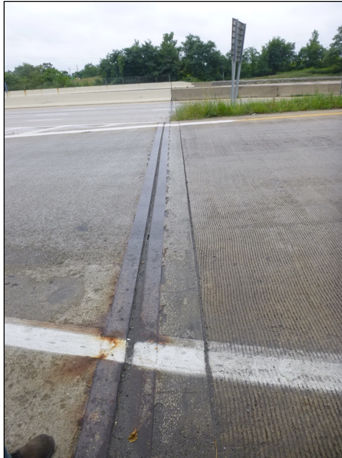
Picture #24: Typical full width spalling on westbound abutment expansion joint headers, looking south along ramp C-7.
