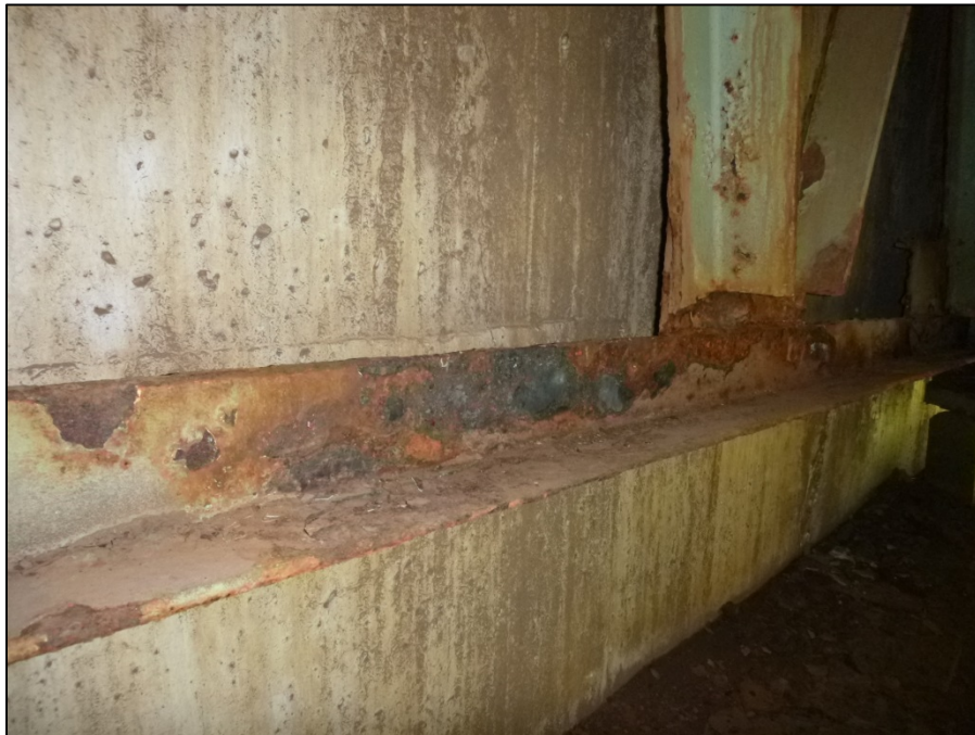
Picture #32: End crossframe in span 25R, between girders X and Y, looking east. Up to 50% section loss on bottom chord angle.
