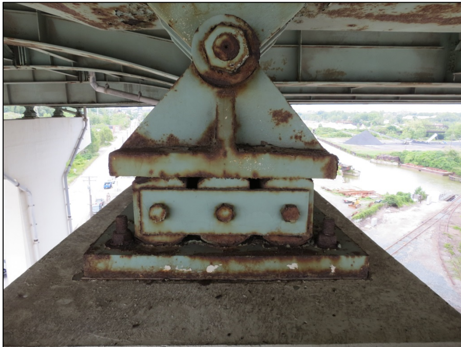
Picture #38: Surface corrosion on girder J roller bearing at pier 9R, looking north.
