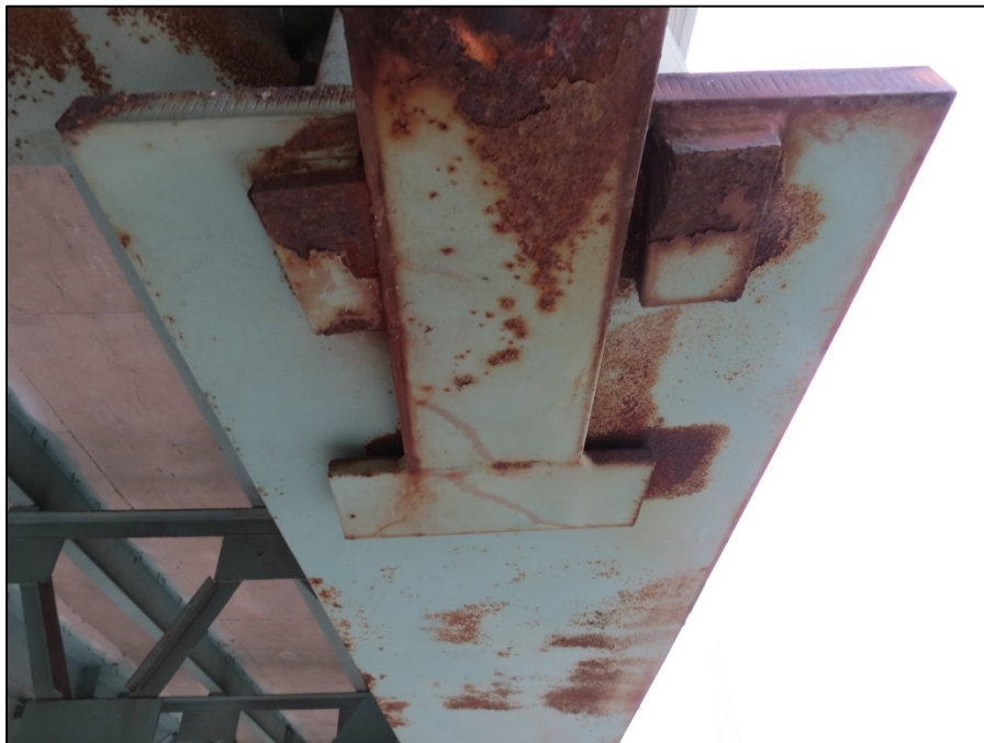
Picture #26: Shear key rubbing on south keeper plate of girder A in span 9L, looking west.
