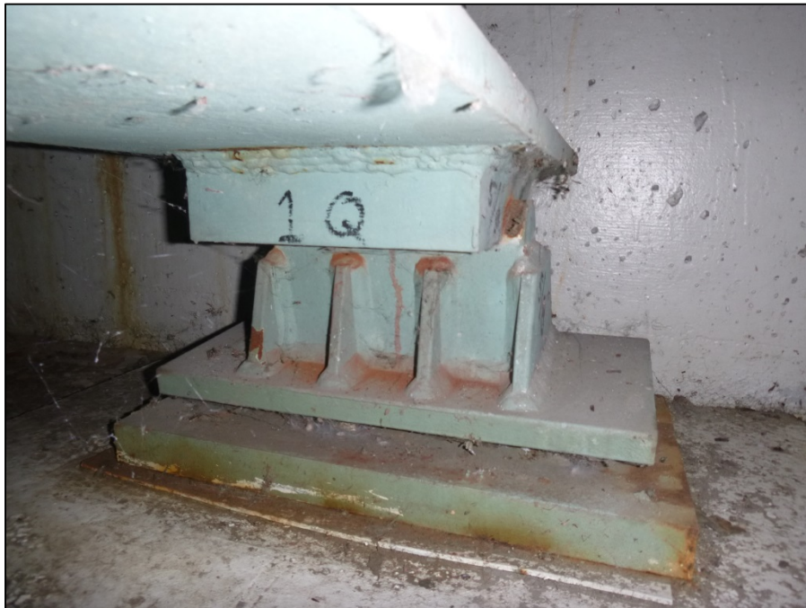
Picture #40: West abutment rocker bearing 1-Q offset 13/16" north, looking west.
