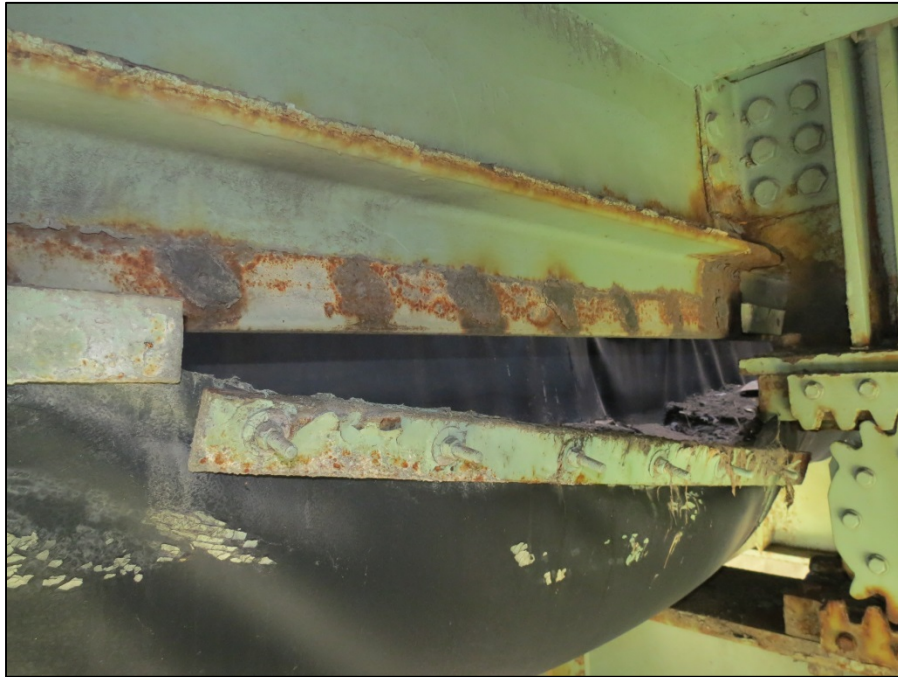
Picture #21: Failed neoprene trough support at roller 5R, looking northwest.
