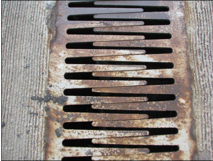
Picture #8: Finger joint in span 6 misaligned transversely, looking south.
