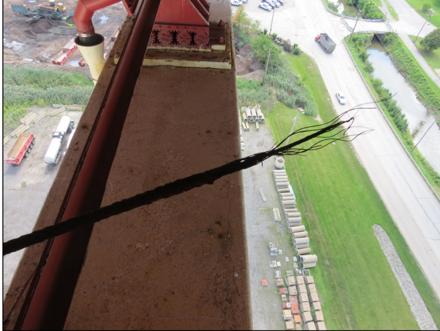
Picture #20: After safety cable snapped at pier 9, looking south.
