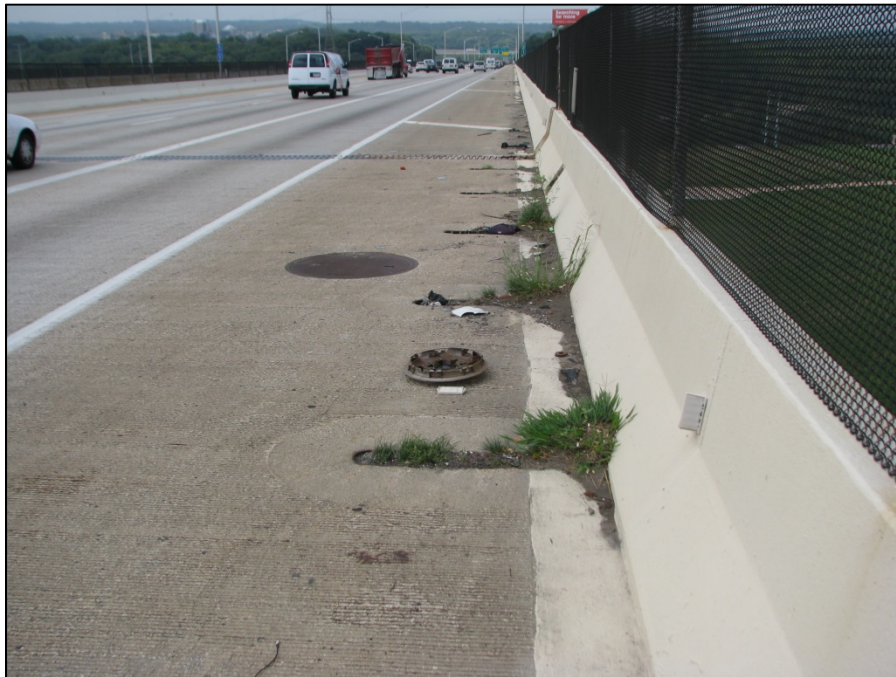
Picture #3: Typical debris in scupper grates and one plugged downspout along the north parapet at pier 9, looking west.
