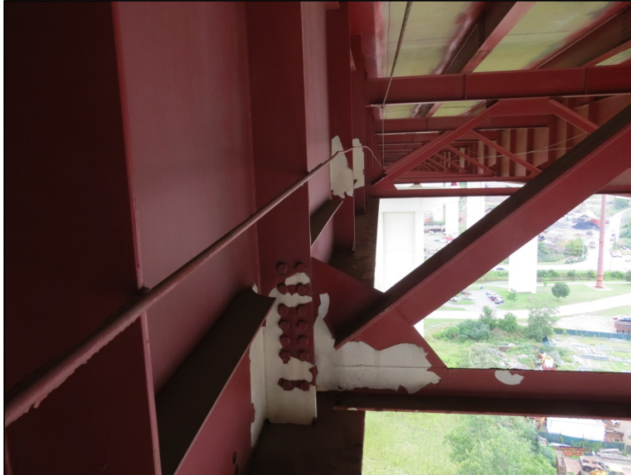
Picture #12: Top coat paint failure on south face of girder B in span 7, looking east.
