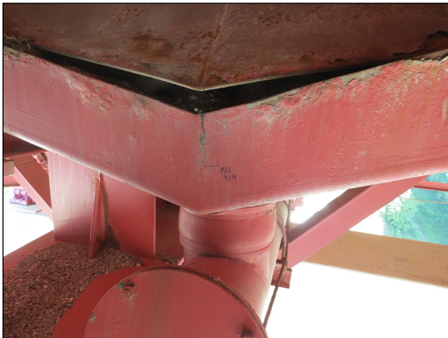
Picture #5: Crack in drainage trough next to south face of girder B in span 12, looking east.
