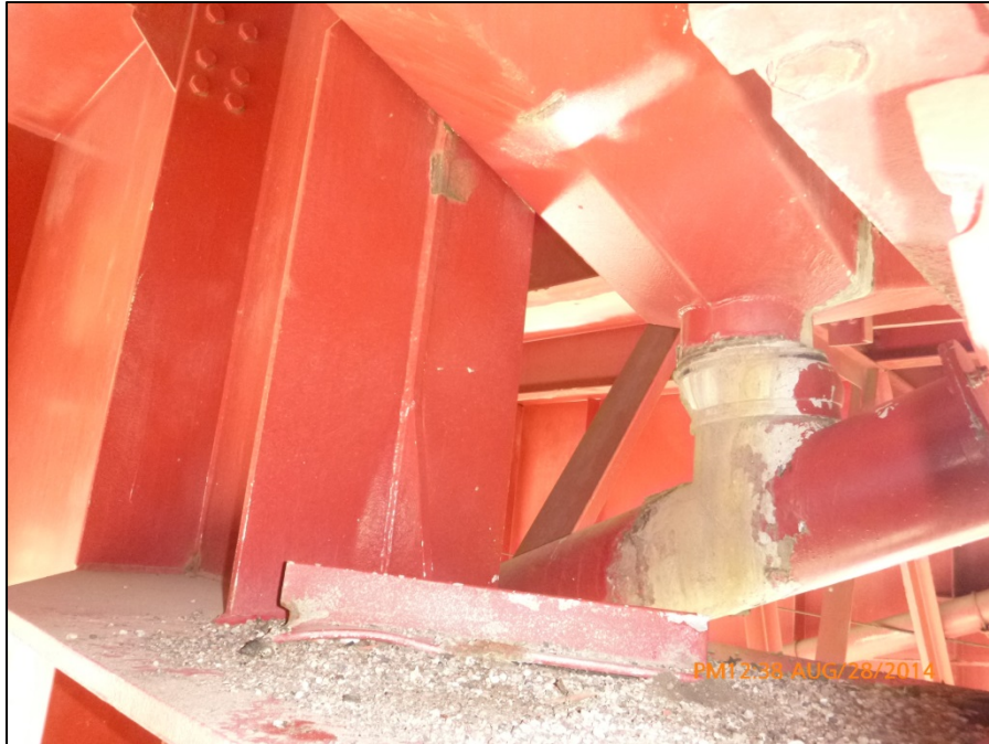
Picture #6: Broken drainage trough support angle next to girder B in span 9, looking east.
