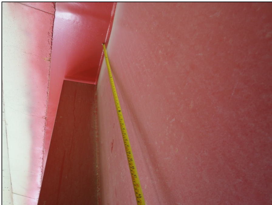
Picture #9: 1” bow near top of girder B web, west of span 14 floorbeam 1, looking north.
