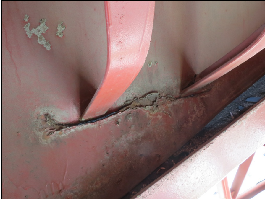
Picture #4: Support angle punched through drainage trough flashing next to south face of girder B in span 9, looking east.
