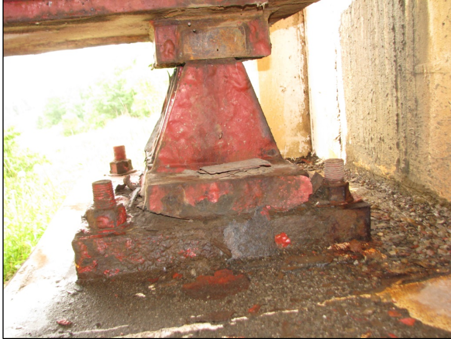
Picture #11: Dirt and deterioration on forward abutment girder A bearing, looking north.
