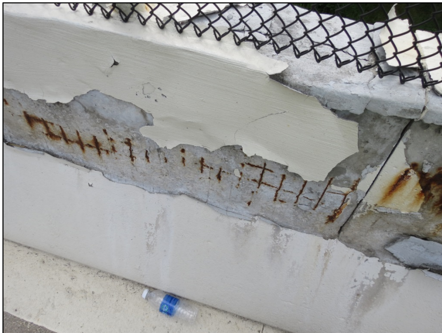
Picture #2: South parapet repairs and sealing failing in span 15, looking south.
