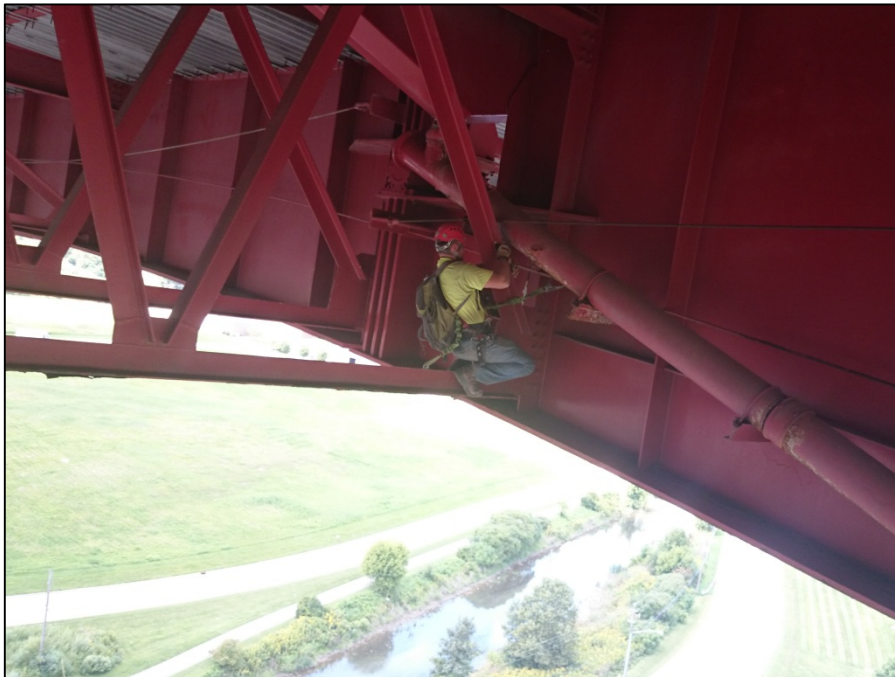
Picture #19: Inspector passing under deteriorated cable prior to snapping, looking north.
