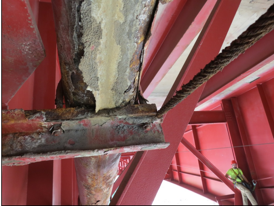
Picture #18: Deteriorated safety cable along south face of girder B near pier 9 prior to snapping, looking east.
