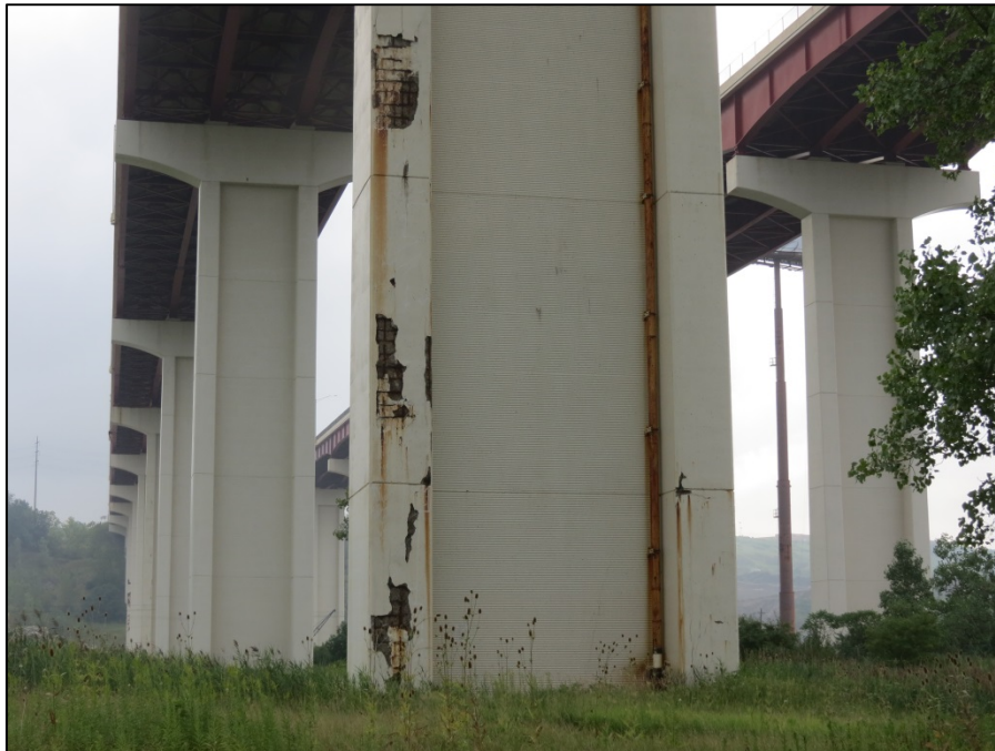
Picture #13: Deterioration on west face of pier 6, looking east.
