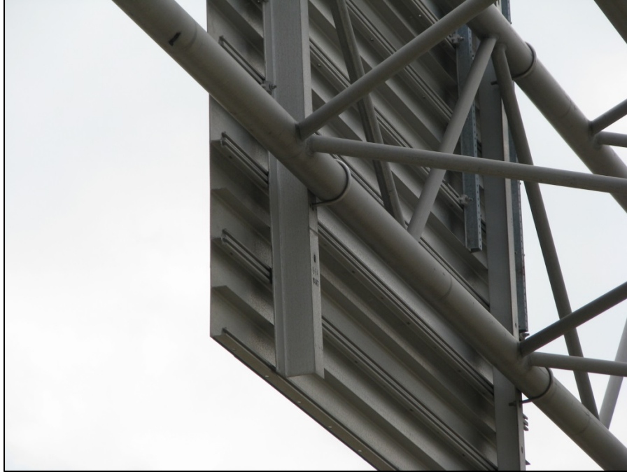
Picture #16: Sign clips missing from bottom half of overhead sign in span 11, looking south.
