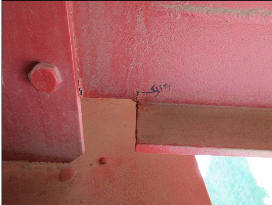
Picture #10: Active 3/4-inch cope crack on floorbeam 10 at connection to south face of girder B in span 12, looking east.
