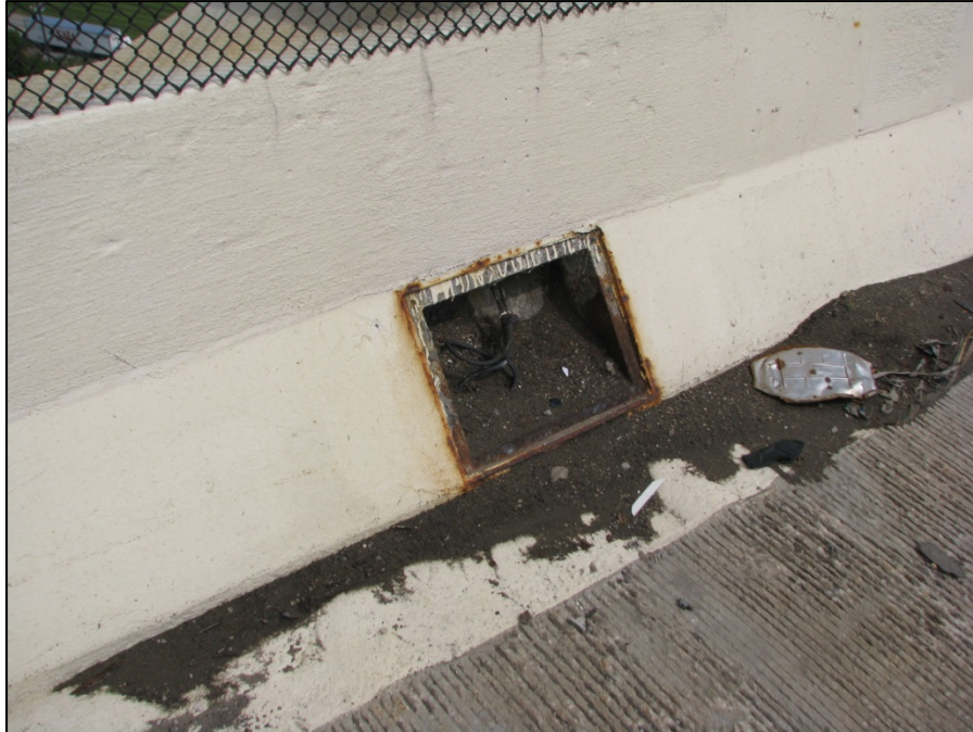
Picture #17: Missing electrical junction box cover in north parapet in unit 3.
