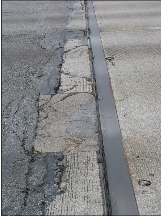
Picture #15: Top of the forward abutment backwall breaking up in lane 1N and 2N, looking south.
