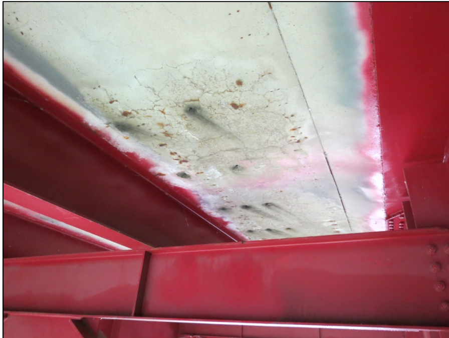
Picture #1: Leaking and cracks around holes drilled through deck in span 2, center bay, near floorbeam 8.
