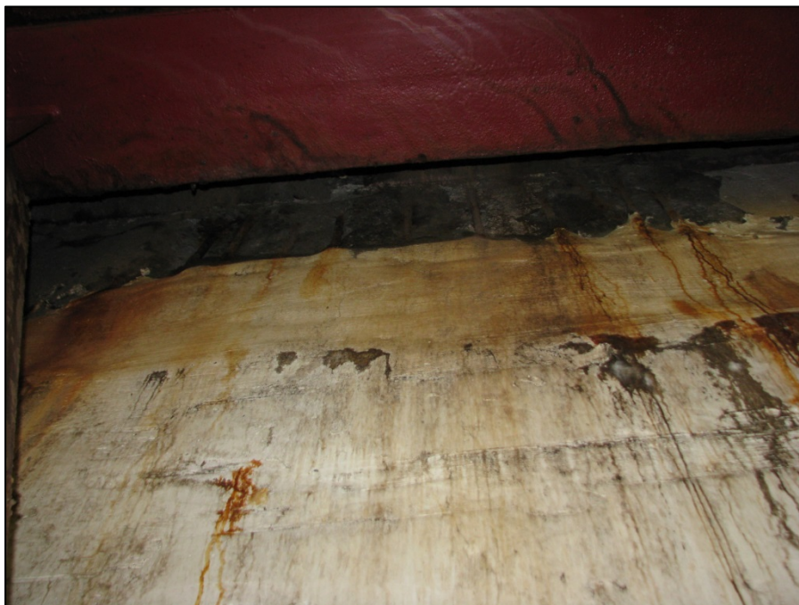
Picture #14: Top 3 feet of forward abutment backwall not patched and some patches already failing, looking east.
