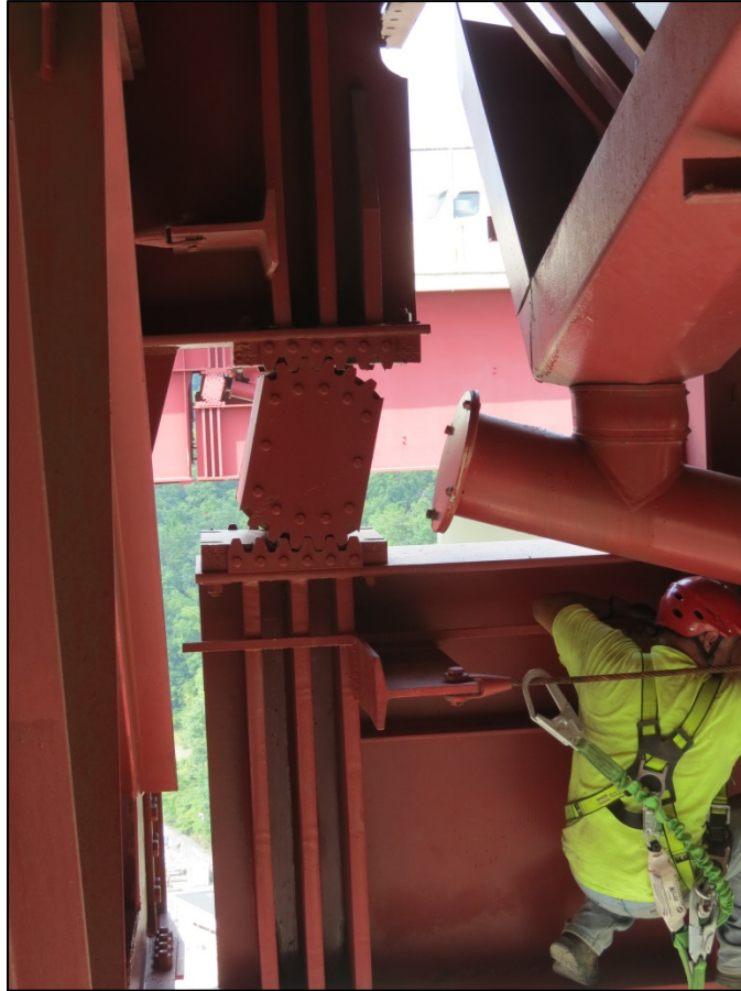
Picture #17: Girder E hinge rocker near pier 12 tilted 12° East at 90°F.
