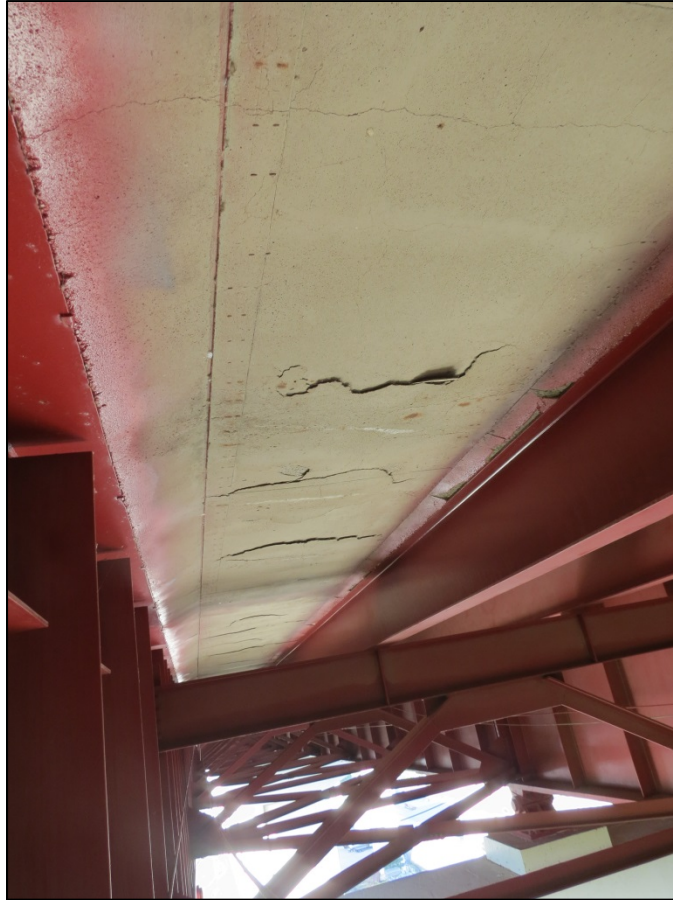
Picture #2: Typical deck cracks and delaminations in span 15.
