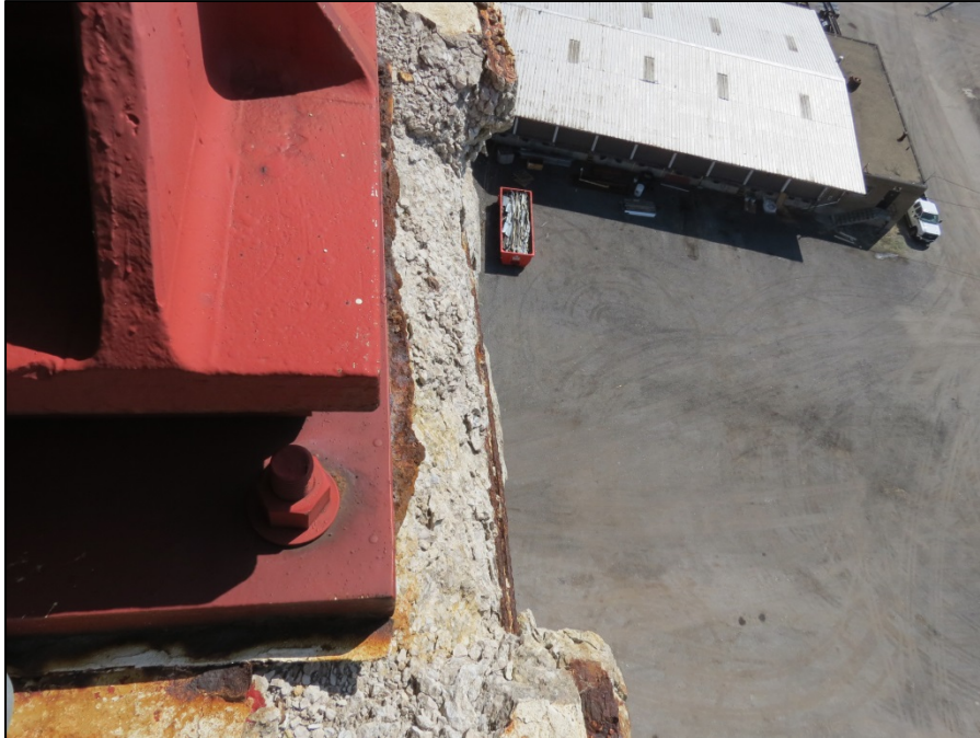
Picture #19: South end of pier 4 cap deterioration undermining edge of girder H bearing.
