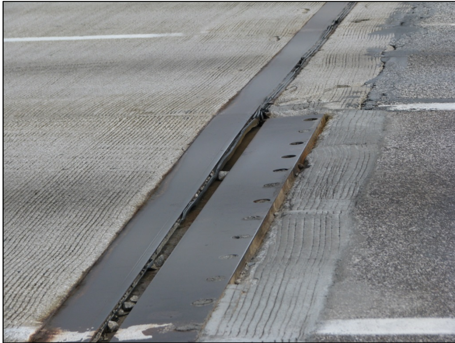
Picture #8: Forward abutment joint armor breaking up in lane 2. Banging with traffic.
