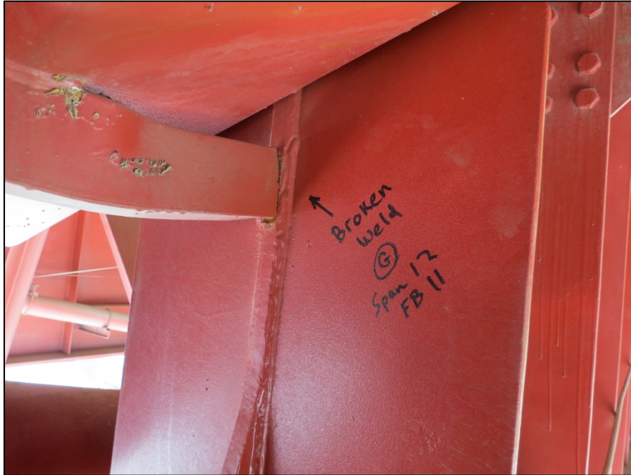
Picture #4: Cracked weld connecting drainage trough support angle to girder G in span 12, looking north.
