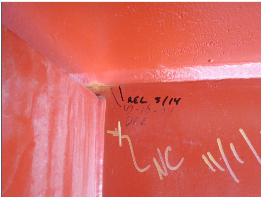
Picture #11: Active 3.25" crack on south face of girder G, span 6.
