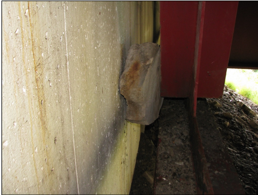
Picture #14: Large chunk of backwall concrete wedged between center bay end floorbeam and the forward abutment backwall, looking south.
