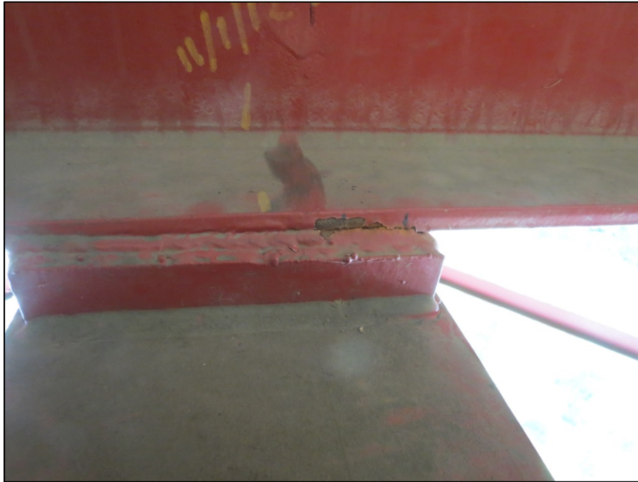
Picture #13: Cracked stringer 11 welded connection to floorbeam 8 in span 3, looking south.
