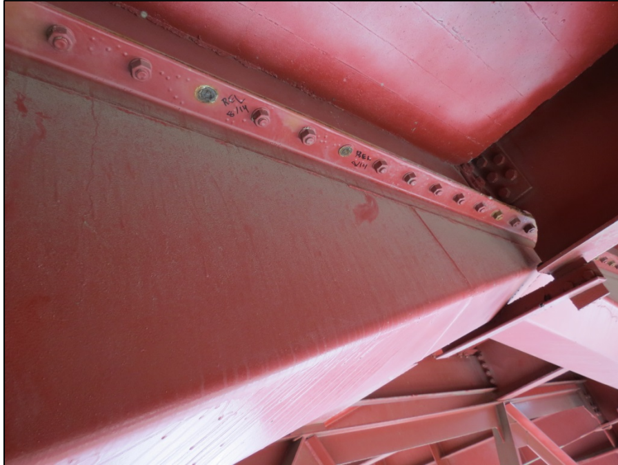
Picture #5: Two broken bolts connecting drainage trough to joint support armor between girders E and F near pier 12, looking west.
