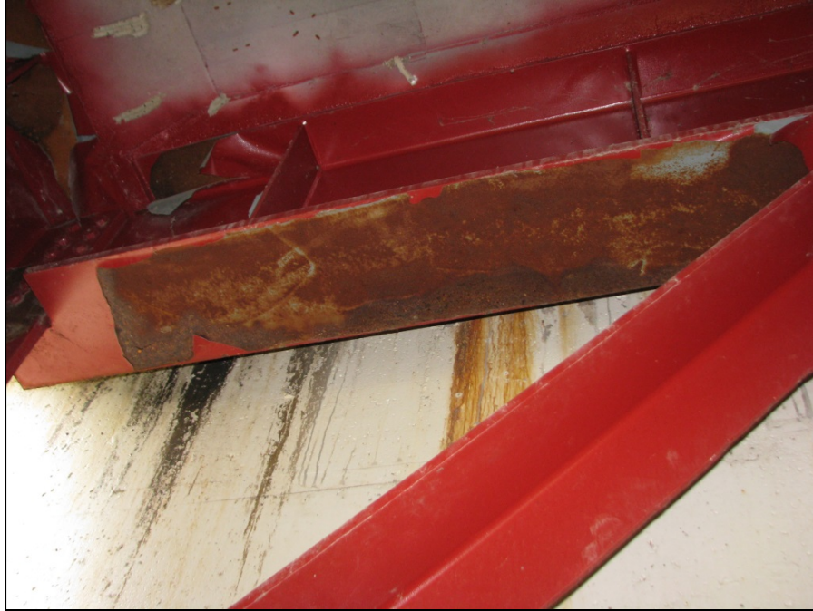
Picture #16: Paint failure on rear abutment end floorbeam near girder H.
