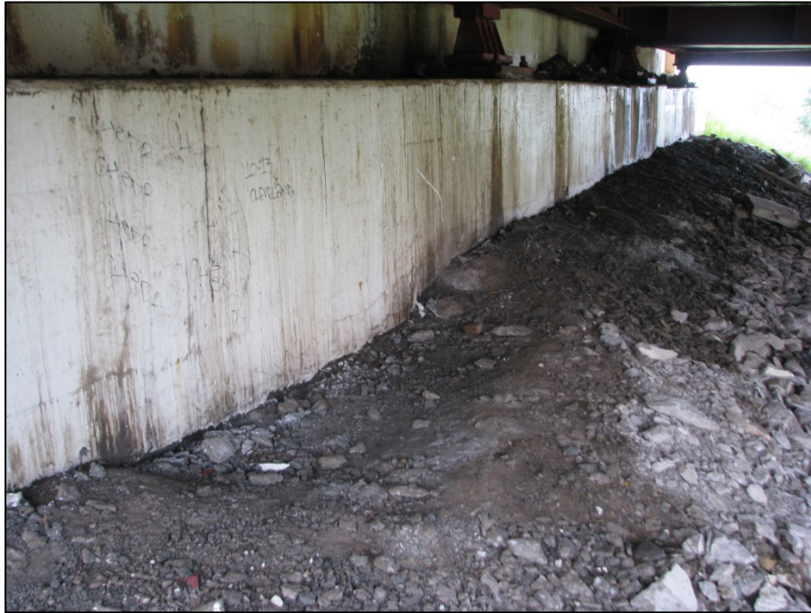
Picture #23: Top of forward abutment slope protection never restored after 2013 rehab.
