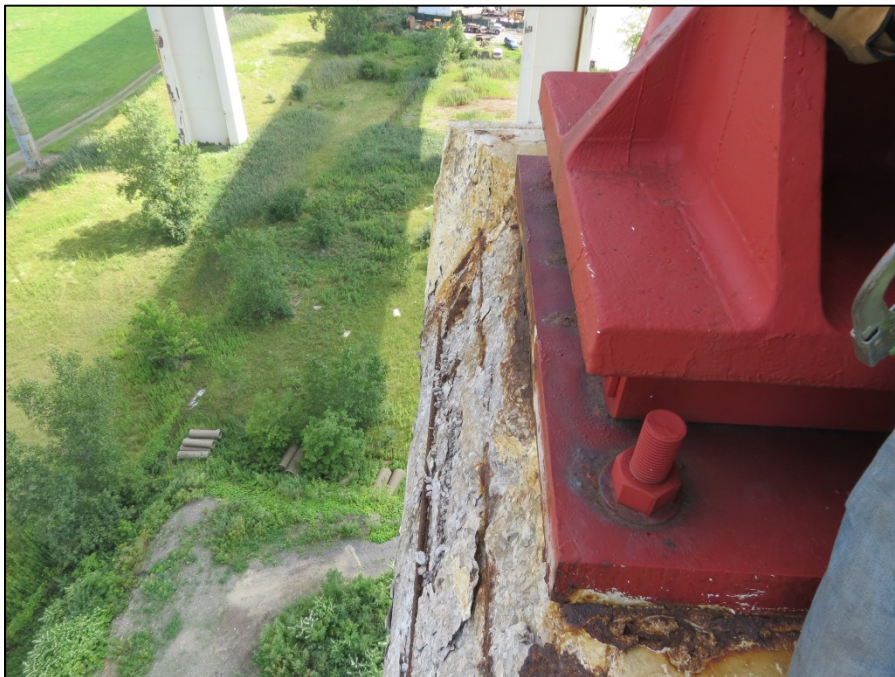
Picture #20: North end of pier 5 cap deterioration undermining edge of girder E bearing.
