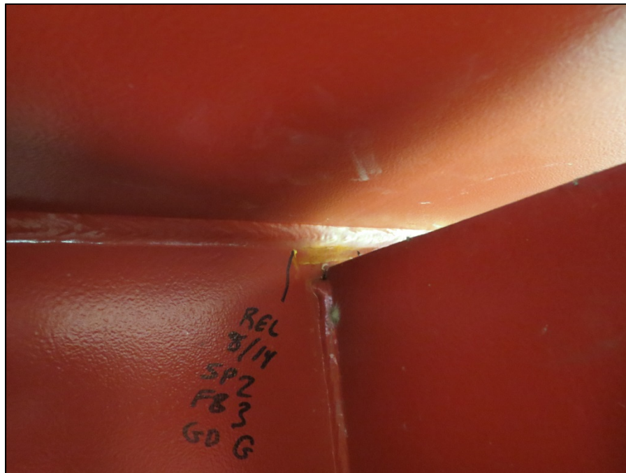
Picture #9: New 2.25” active crack on south face of girder G, span 2.
