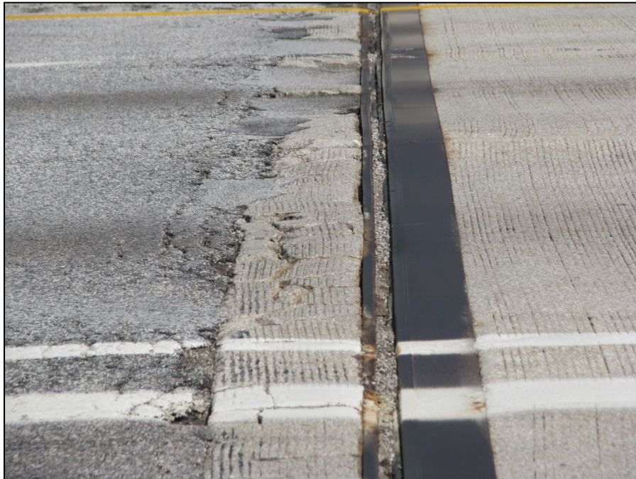
Picture #7: Rear abutment joint header breaking up in lane 3, looking north.
