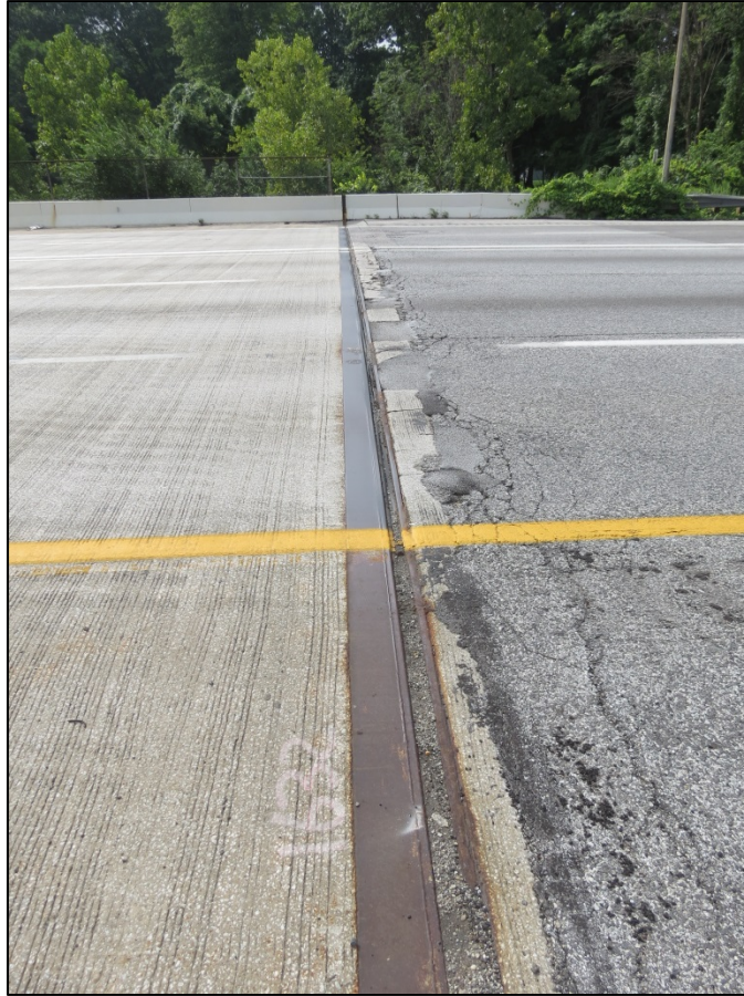
Picture #6: Rear abutment joint header breaking up, looking south.
