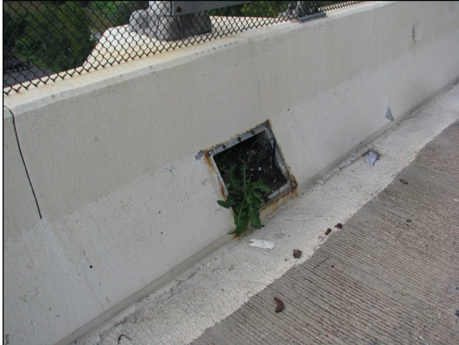
Picture #24: Electrical junction box cover missing from south parapet in span 5.
