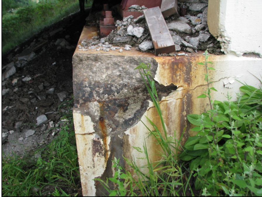
Picture #18: Spalls and deterioration at south end of forward abutment. Note debris on seat.
