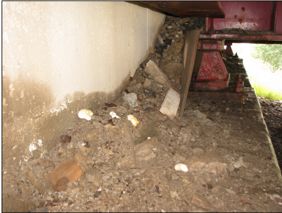
Picture #15: Forms and concrete debris blocking expansion of girder G rocker at forward abutment, looking south.
