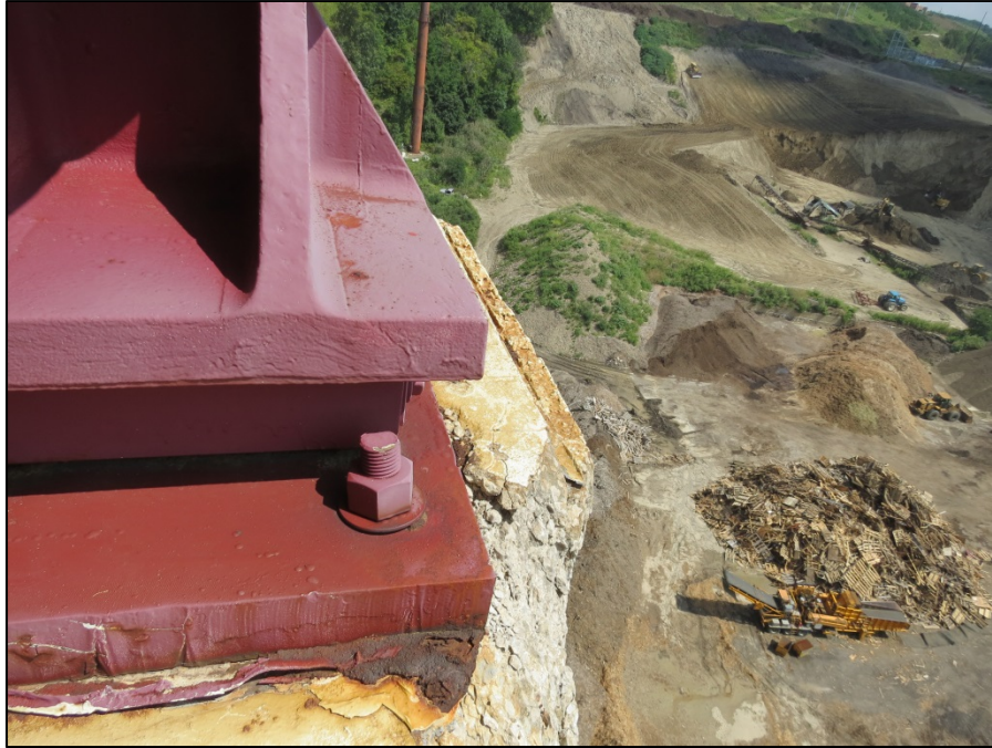
Picture #21: South end of pier 11 cap deterioration undermining edge of girder H bearing.
