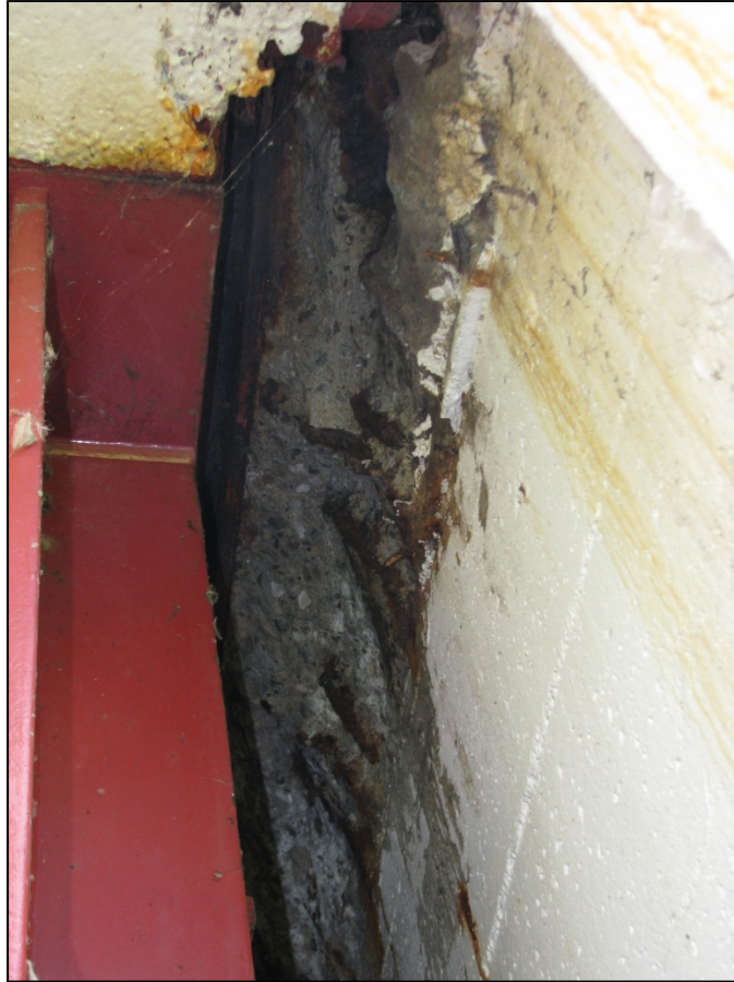
Picture #22: Top of rear abutment backwall continuing to deteriorate behind girder E.
