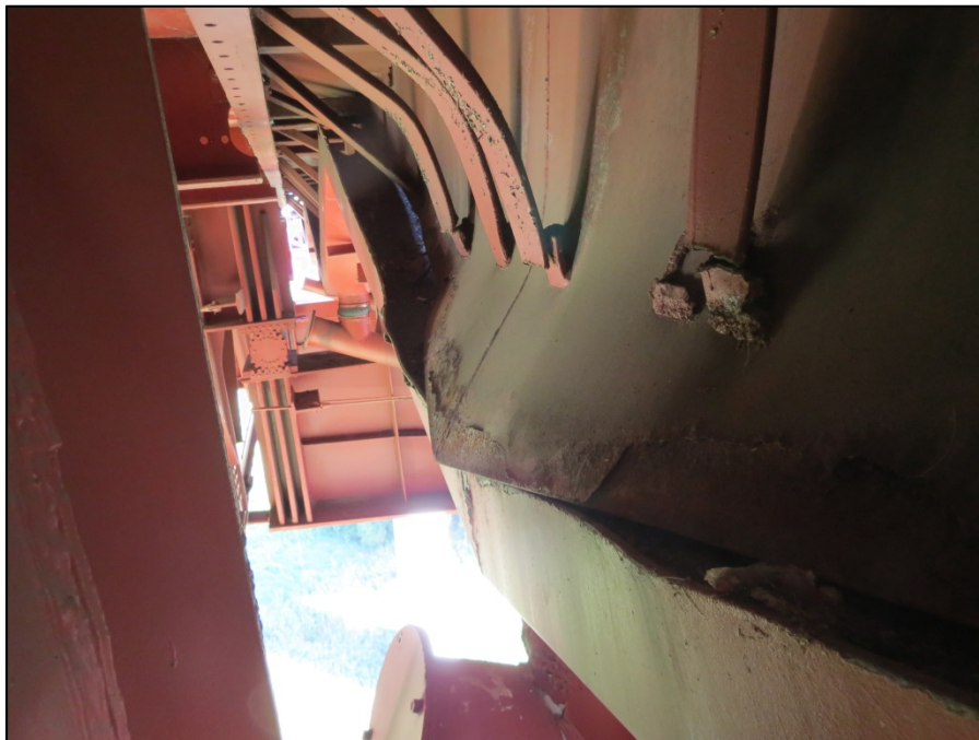
Picture #3: Steel flashing bent out of trough. Support angles bent and broken Looking north from girder G in span 3.
