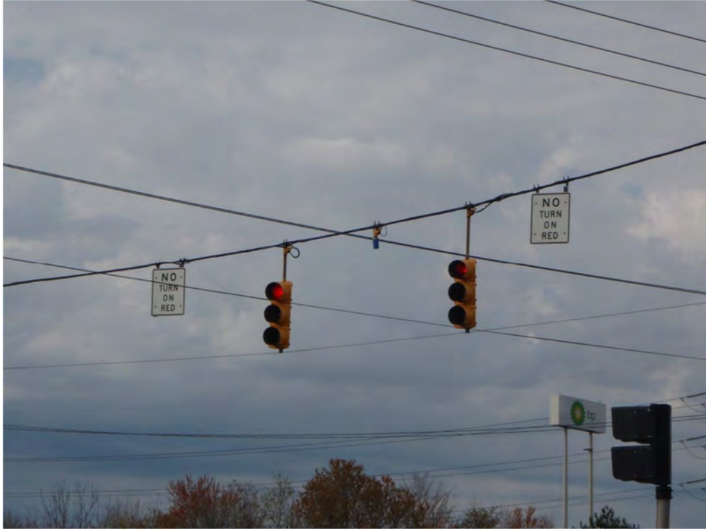
Photo 23. S.R. 82 and I-71S Signal Head from ramp
