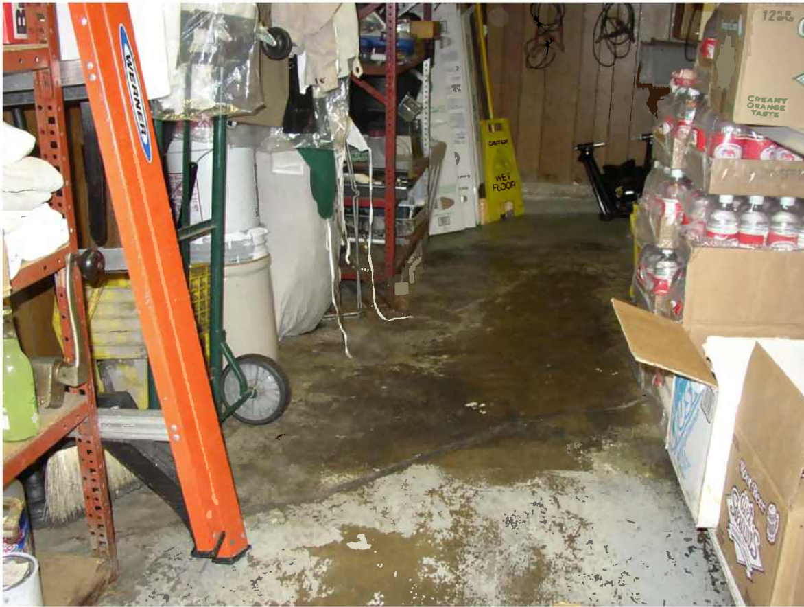
Figure 8: 1201 University Avenue (Sokolowski's University Inn). Photo is taken from inside looking at the north-west corner of the building. This photo illustrates settlement that occurred approximately 5 years ago. The maximum vertical displacement is at least 9-inches (BBCM, 2005b).
