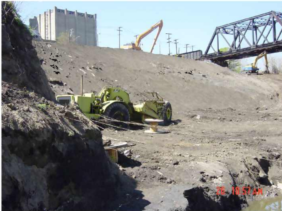
Figure 3.1: Pictures showing the failed sheet pile wall.
