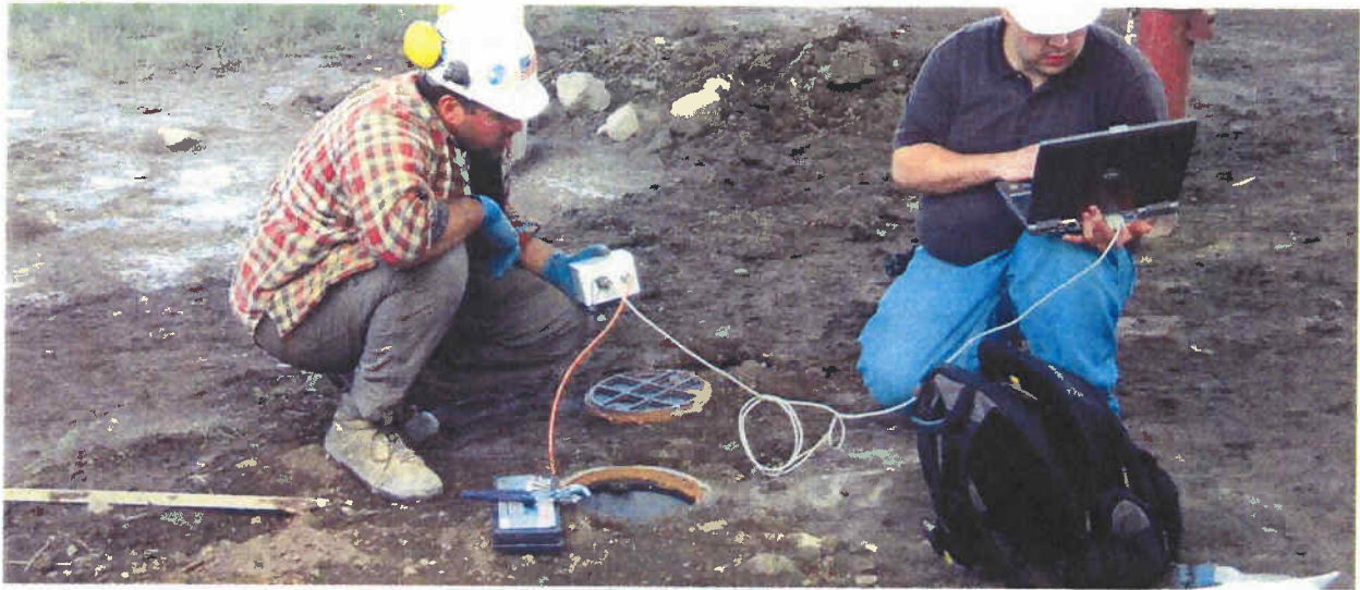
a) BBCM personnel performing an initial reading of a vibrating wire piezometer.
