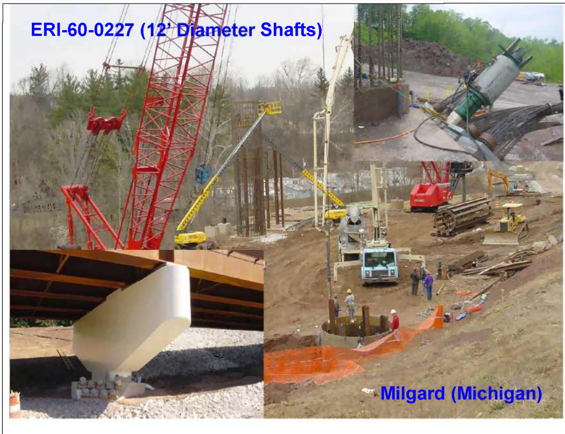
Figure 9.6: Example of a drilled shaft tied back for resistance of lateral soil forces
