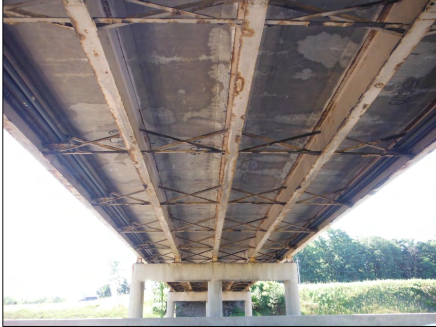
Photo 4: Looking east over the southbound lanes at deck spalling.
