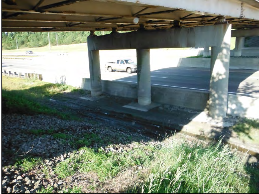
Photo 1: Typical view under the bridge looking at pier 3. Note the south column deterioration.
