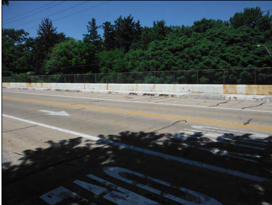
Photo 3: Looking at the north railing and deteriorated curb near the center of the bridge.
