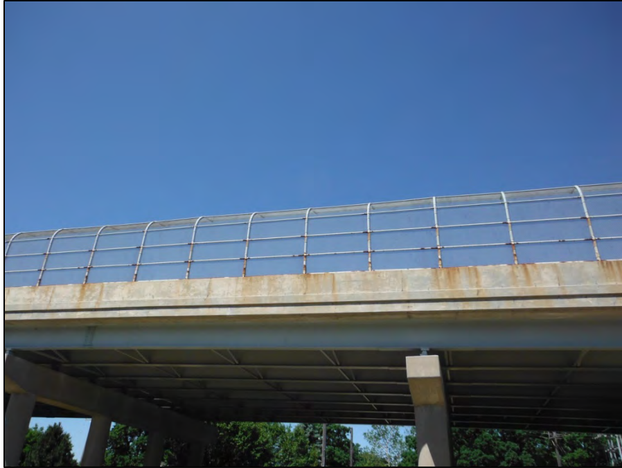
Photo 1: Typical view of east fence and parapet. Note fence post and rail rusting and the staining of parapet.
