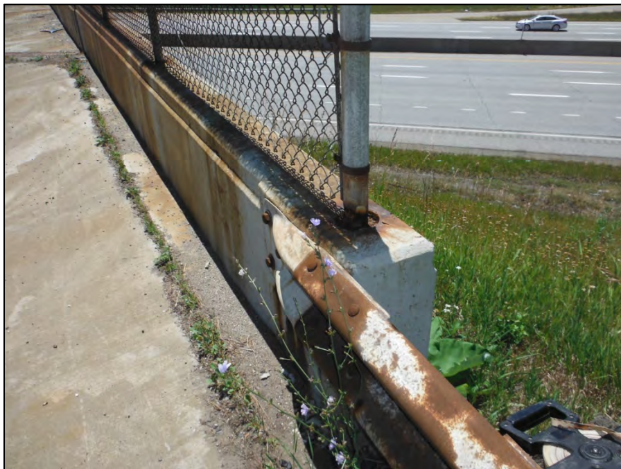
Photo 2: Looking at northwest corner of east railing. Note the fence post pipe sleeves embedded in the concrete railing and no base plates.
