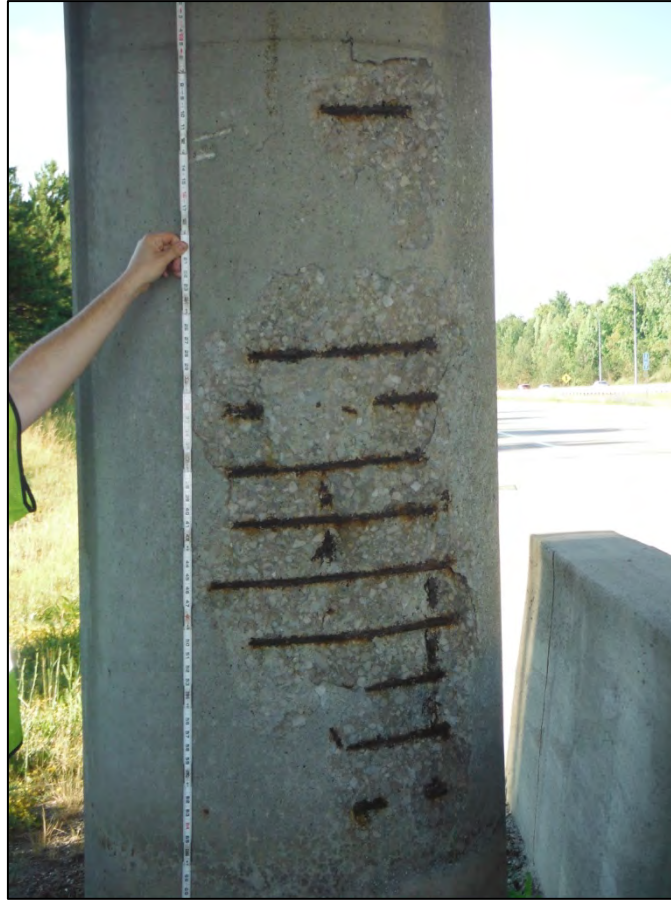
Photo 5: Pier 3 south column spalling and deterioration
