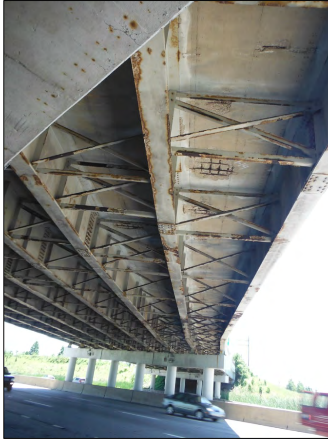
Photo 3: Looking south over westbound lanes at deck delamination and the exposed bottom mat of reinforcing steel.
