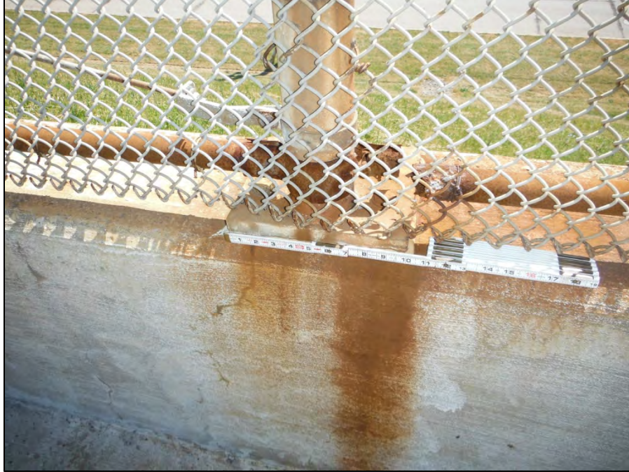
Photo 3: Typical fence deterioration that is primarily located in the lower portion of the fence.
