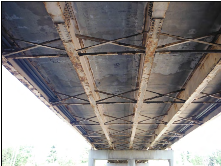
Photo 2: Looking west over the northbound lanes at deck spalling/delaminations.
