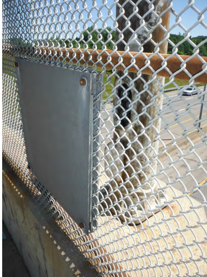
Photo 4: Light pole on east parapet (there is also a light pole on the west parapet).
