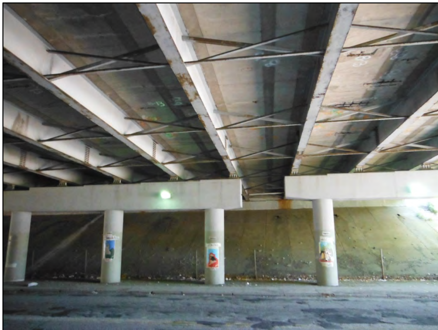
Photo 2: Typical view under the bridge looking east under center of eastbound lanes.
