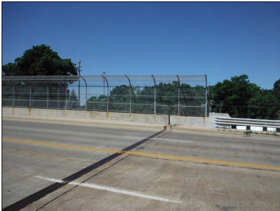
Photo 2: Looking west at north abutment joint. Note the deflection of fence and horizontal rail members due to bridge expansion.
