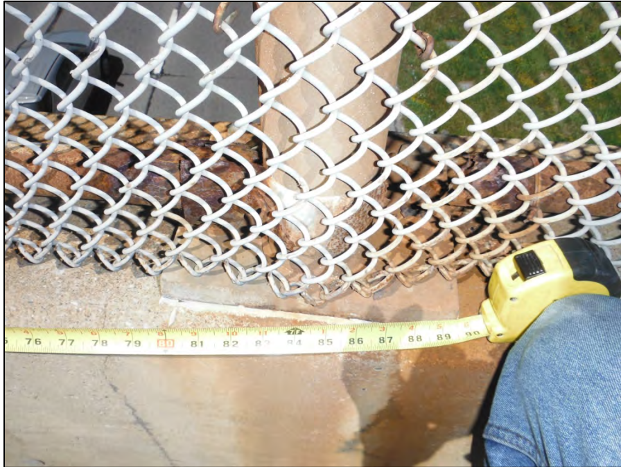
Photo 1: Typical view of east fence and parapet. Note fence post and rail rusting.
