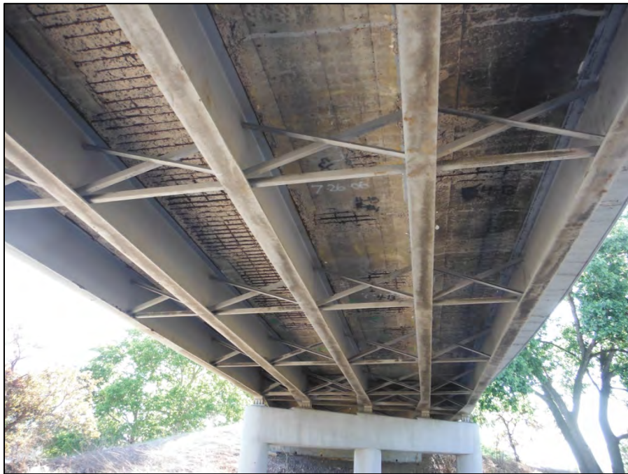
Photo 2: Looking east over the three lane north/west bound ramp at the deck spalling.
