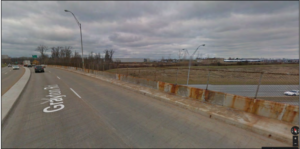
Photo 1: Looking north at east fence and railing. Note rusty fence, railing cracking and previous patching.
