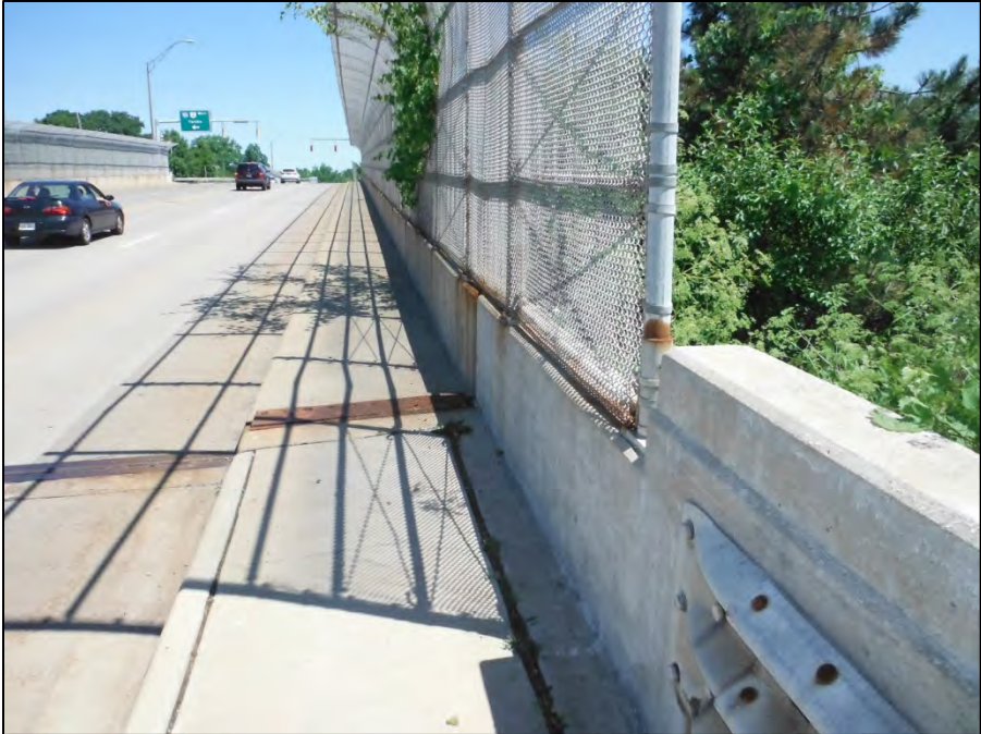
Photo 3: Looking north along east sidewalk and railing.
