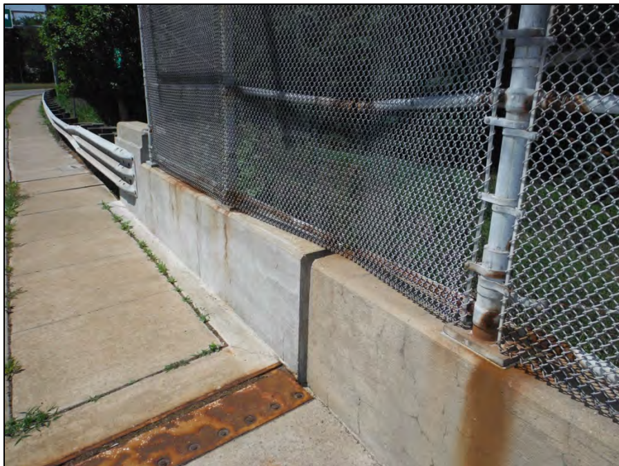
Photo 2: Looking at north abutment joint west railing. Note the deflection of fence and horizontal rail members due to bridge expansion.
