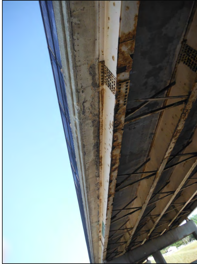
Photo 3: Looking west over the northbound lanes at deck spalling under the south fascia. The loose material should be removed, but it may be impractical to install a timber subdeck outside of the beams (north side fascia is in better condition does not appear to be a problem).
