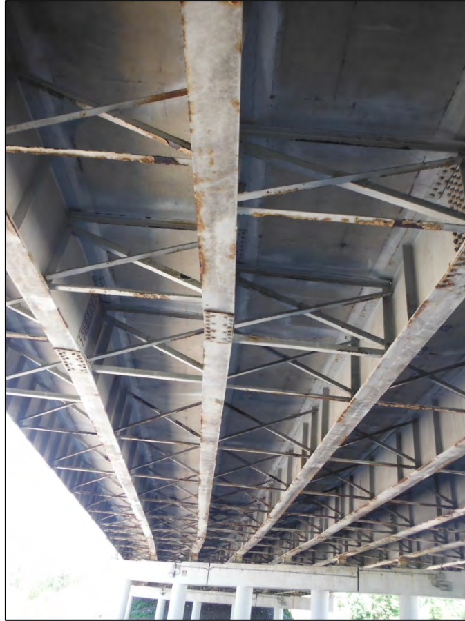
Photo 4: Looking north over eastbound lanes at deck delamination. Generally, the south end is not in as bad of condition as the north portion of bridge.
