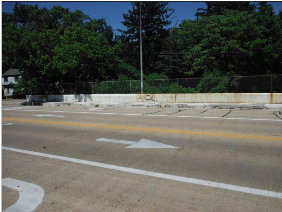
Photo 2: Looking at north railing. Note sidewalk and curb deterioration.
