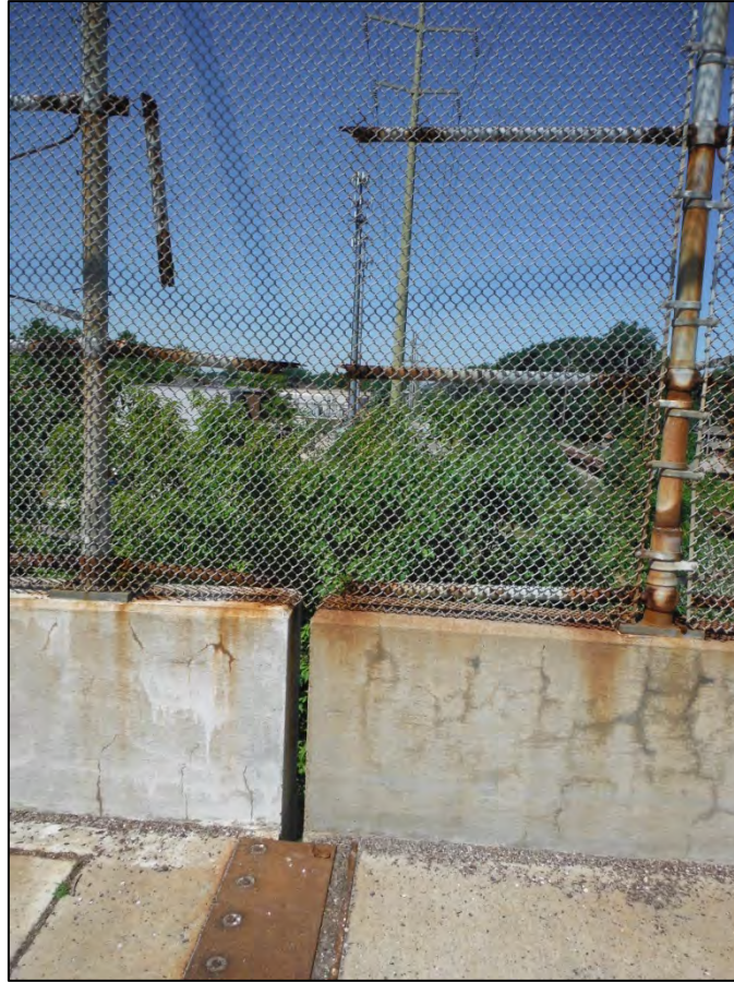
Photo 4: Looking west at south abutment joint at failed fence members.
