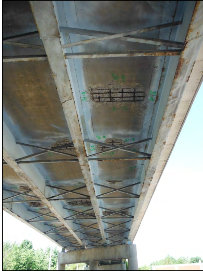
Photo 2: Looking north over the eastbound lanes at deck spalling. This appears to be the worst area.
