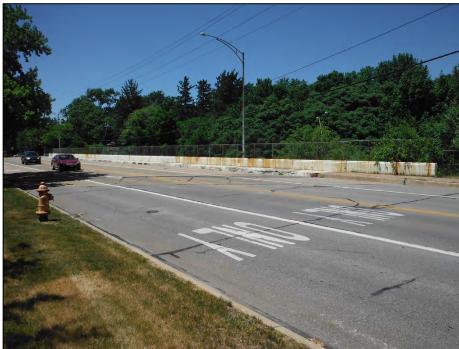
Photo 4: East end of the north railing and sidewalk. This is the worst curb deterioration on the structure.
