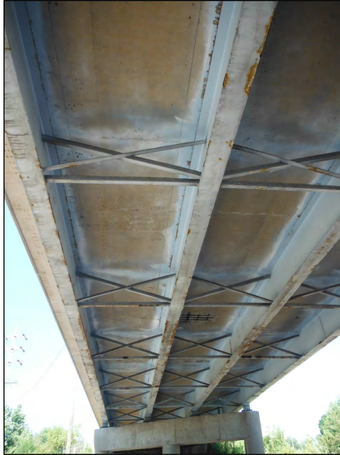
Photo 3: Looking north over the westbound lanes at deck spalling.
