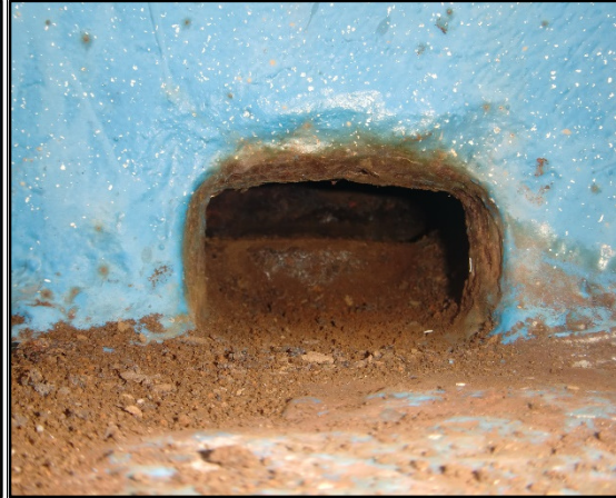
Photo 49B – Steel Casting Blocking Drainage Path.
