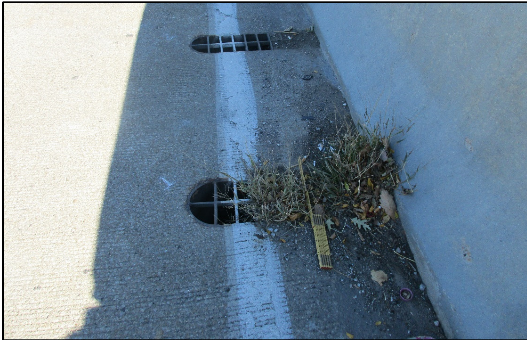
Photo 15 – Typical Partially Clogged Scuppers.
