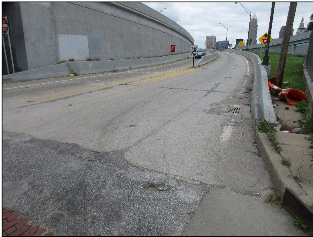
Photo 63 – Typical Approach Slab Condition, W 28 th St. Ramp.
