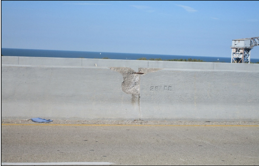
Photo 13 – Spalling of Median Parapet with Exposed Reinforcing, Span 4.
