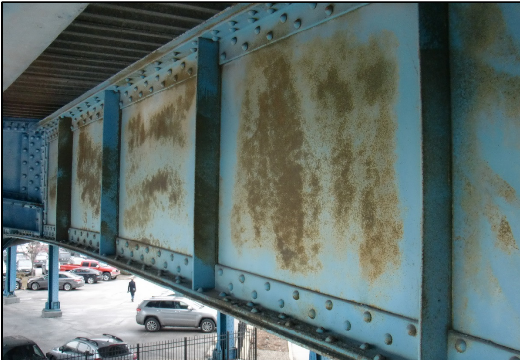
Photo 53 – Common Worn Protective Coating on Girder Web, Lakefront Trestle.
