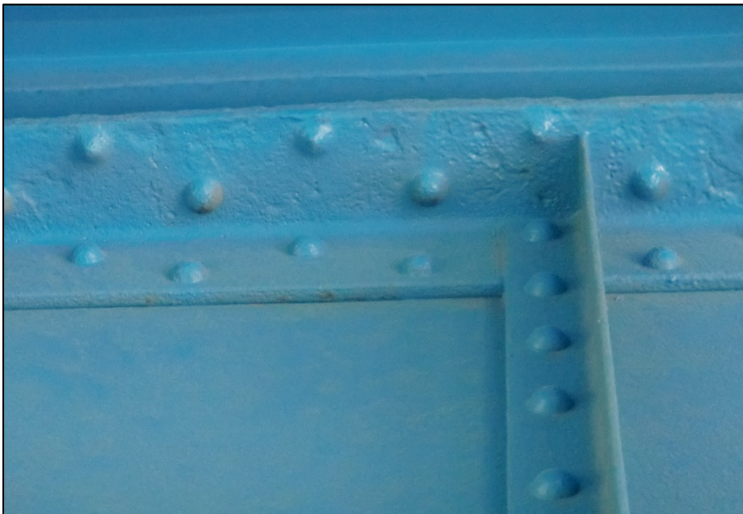
Photo 30 – Typical Top Flange Surface Pitting, Main Truss Floor Beam.
