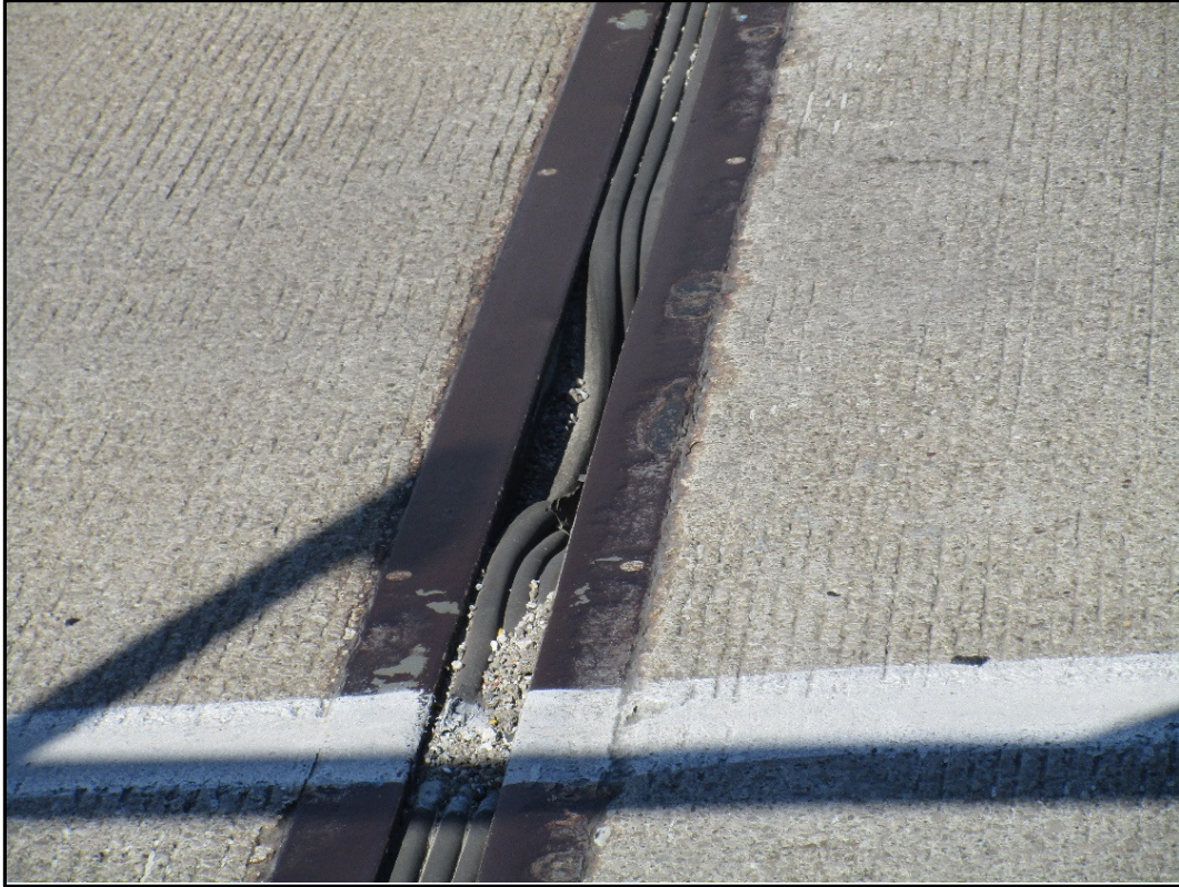
Photo 21 – Detached Joint Seal.
