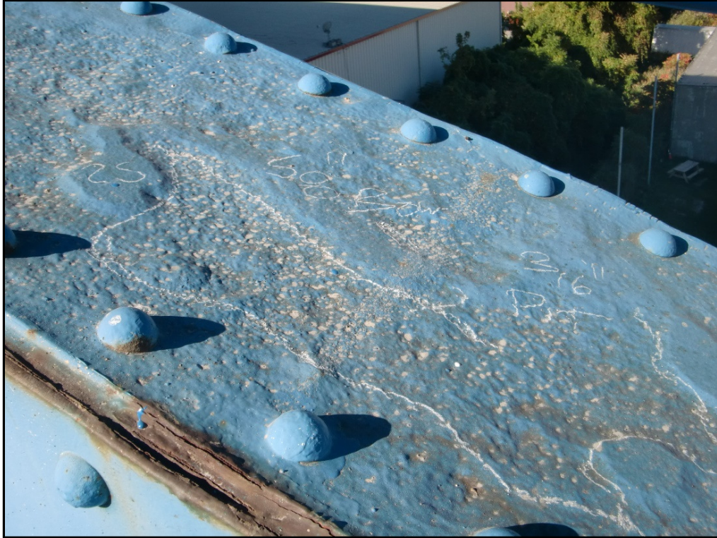
Photo 39 – Typical Pitting of Lower Chord Top Plate.
