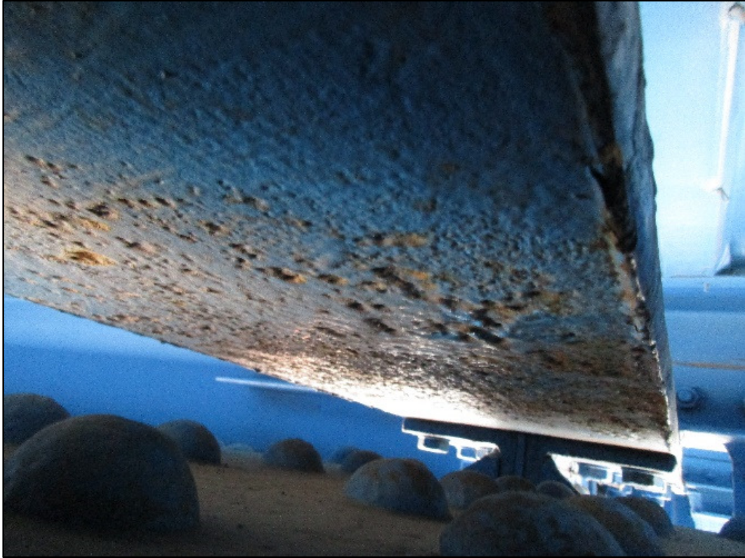
Photo 33 – Typical Top Flange Tension Tie Plate Surface Pitting, Floor Beam, Main Truss.
