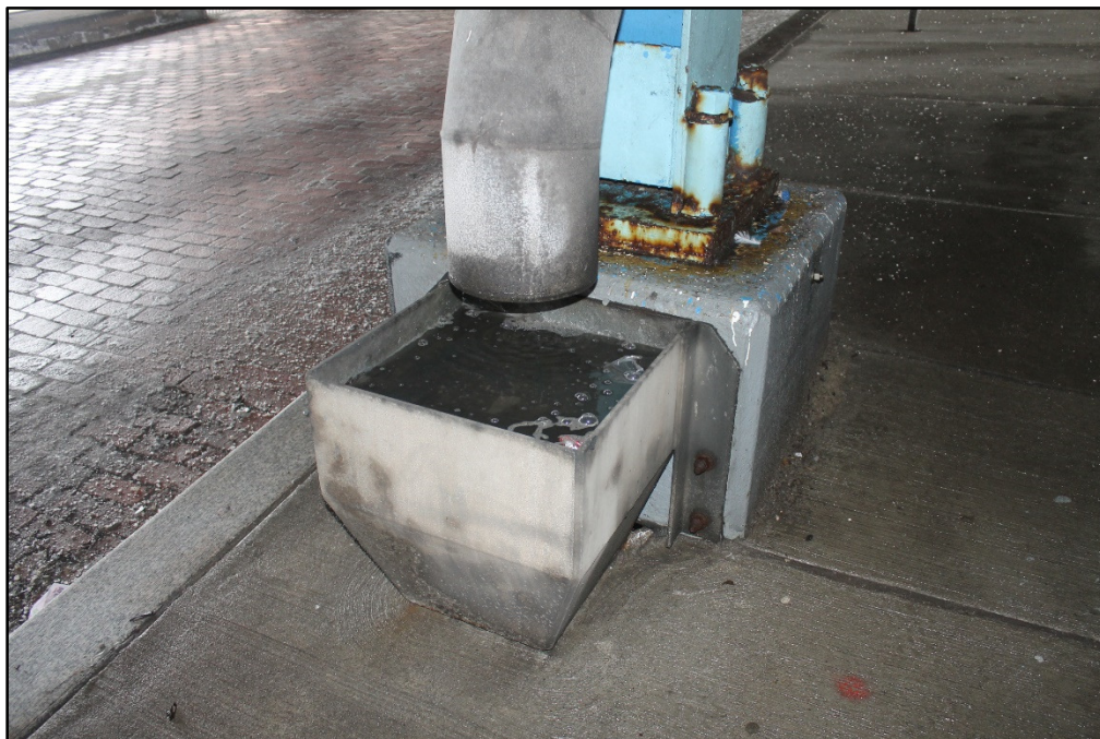
Photo 17 – Typical Clogged Above Ground Collector, Lakefront Approach.
