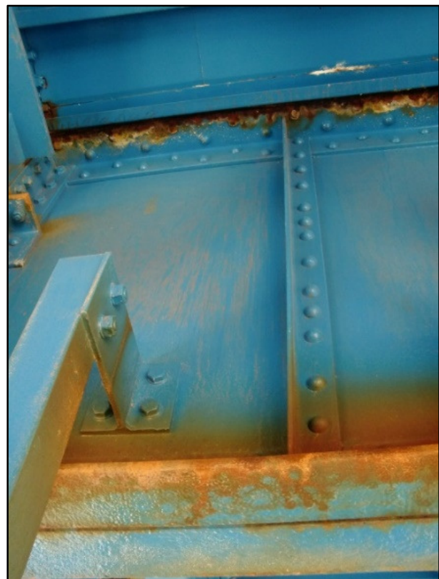
Photo 32 – Typical Rust Staining on Main Truss Floor Beam Under Deck Joint.
