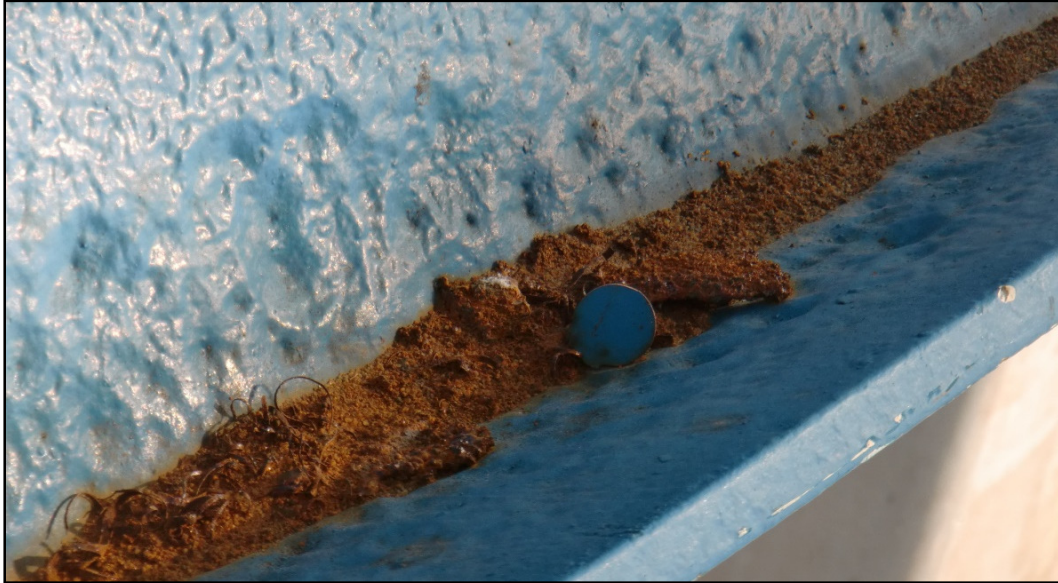
Photo 45 – Common Construction Debris left on Lower Lateral Bracing.
