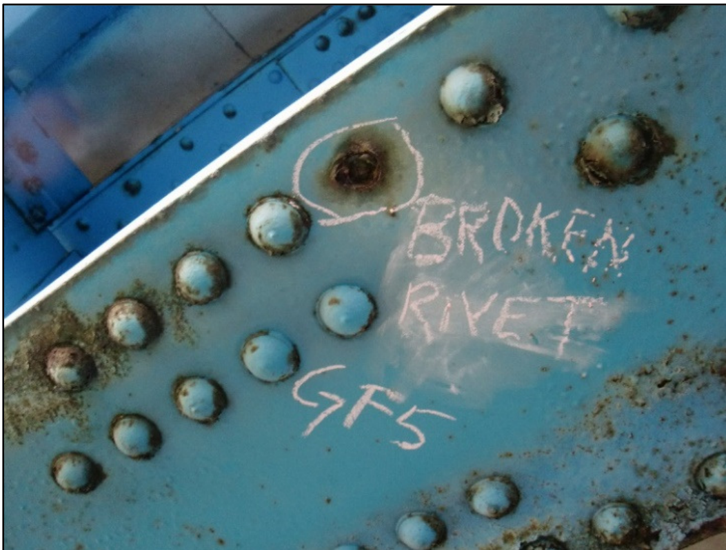
Photo 24 – Broken Rivet, Bottom Flange of Girder GF5, West Approach.
