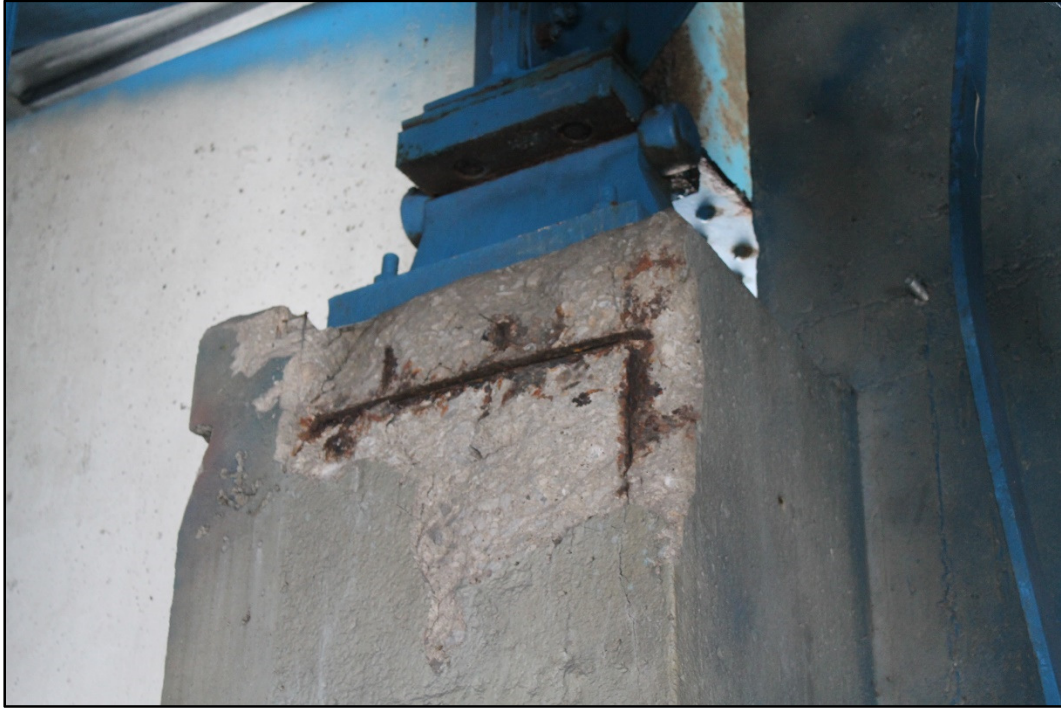
Photo 47 – Spall Undermining of South Bearing Plate, Bent 37.
