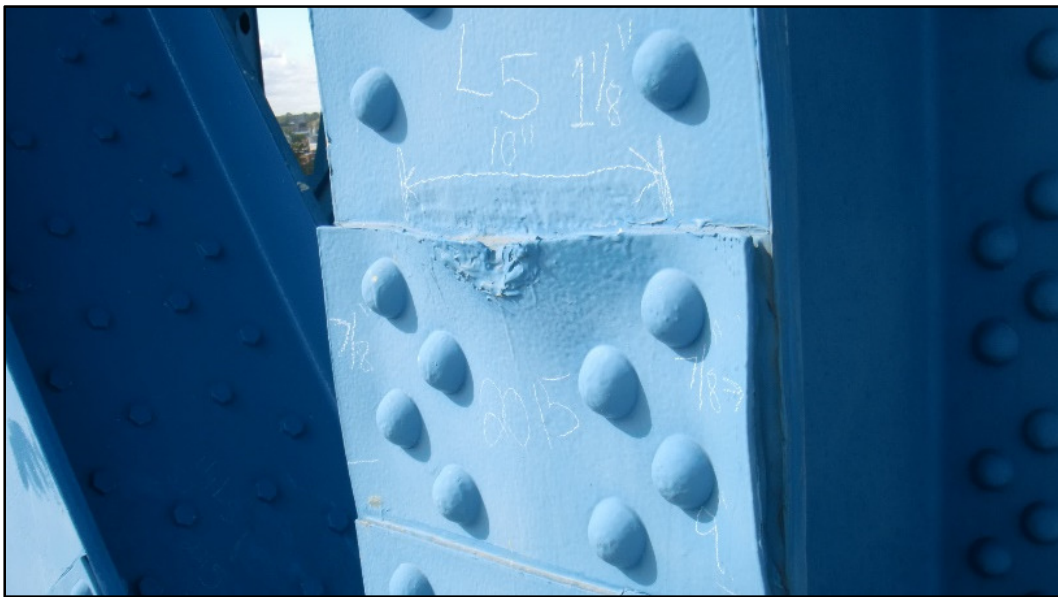
Photo 34 – Typical Pack Rust on Fill Plate, Main Truss Vertical.
