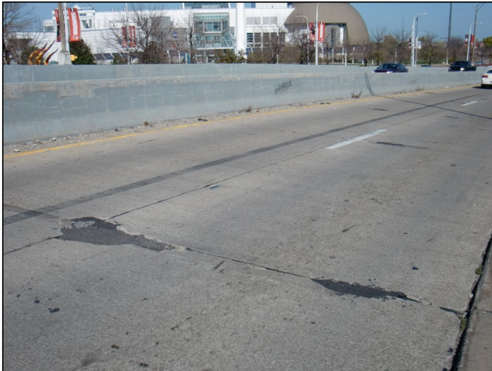
Photo 62 – Patched Spalls in Approach Pavement, East Approach.
