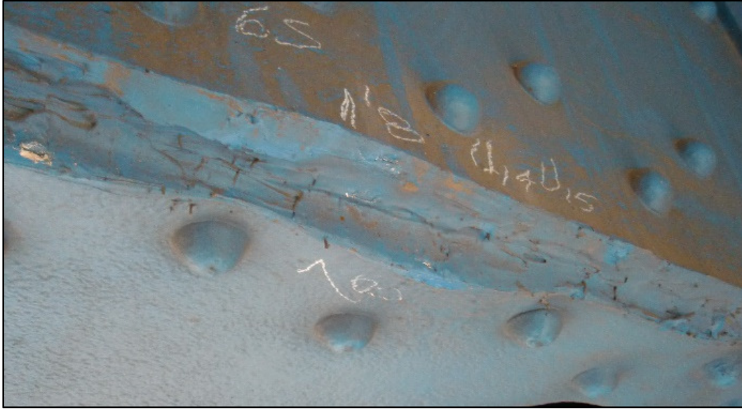
Photo 38 – Typical Pack Rust, South Main Truss, Span 6, U 14 U 15 .
