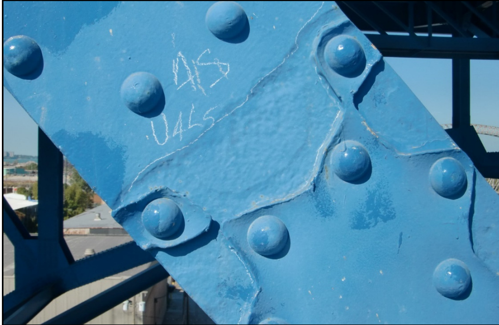
Photo 35 – Typical Fill Plate Section Loss, Main Truss Diagonals.
