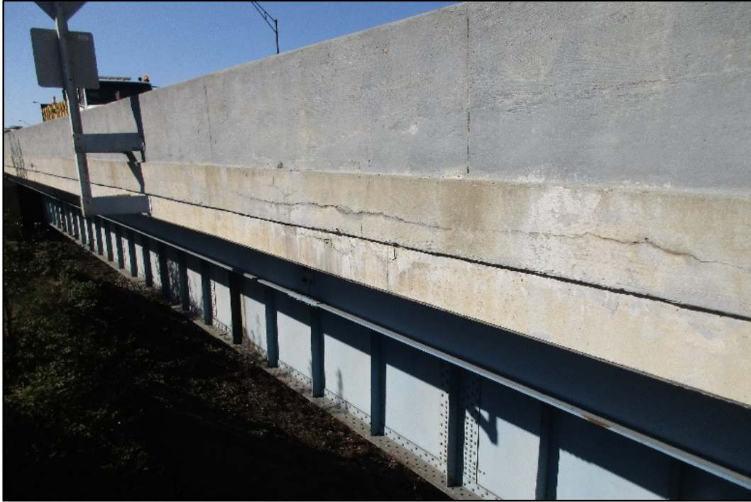
Photo 11 – Early Stage of Railing Deterioration.
