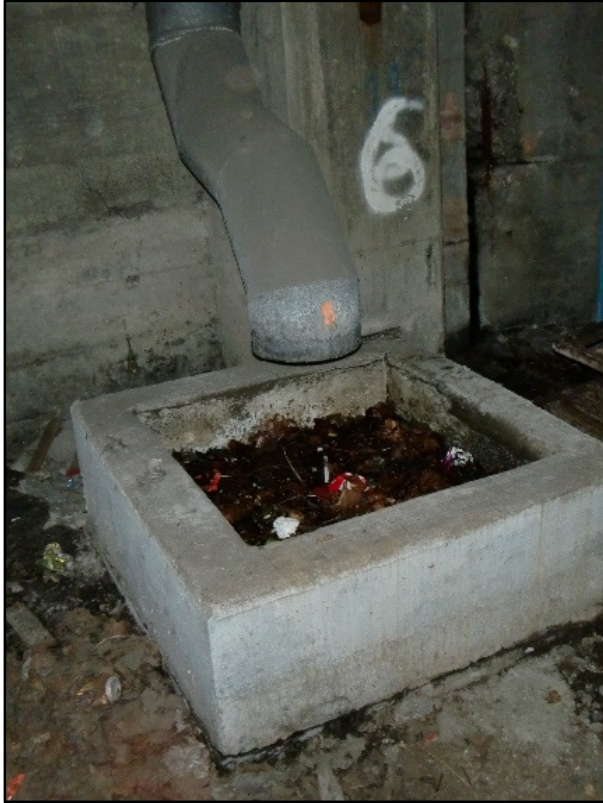
Photo 16 – Typical Clogged Catch Basin.
