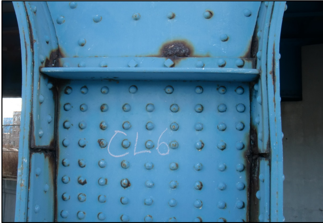
Photo 52 – Typical Local Seam Corrosion, West Approach Superstructure.
