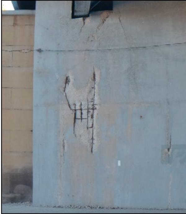
Photo 60 –Typical Mask Wall Deterioration.
