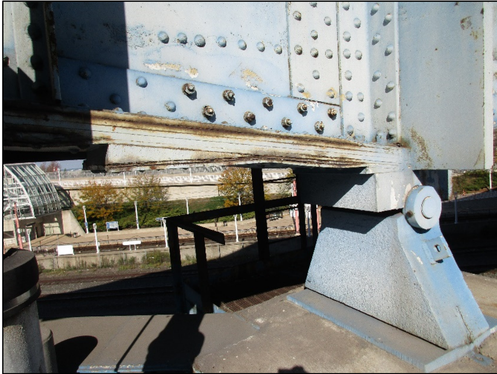
Photo 27 – Typical Pack Rust at Moment Plate, Lakefront Ramp - East Approach.
