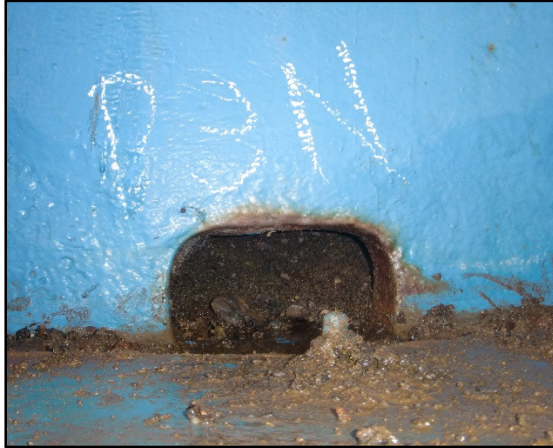
Photo 49A – Typical Debris within Bearing Casting.
