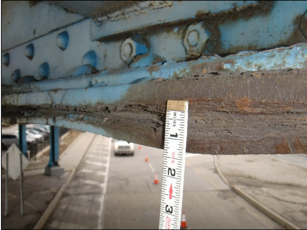
Photo 25 – Typical Pack Rust on Bottom Flange, Lakefront Trestle - East Approach.
