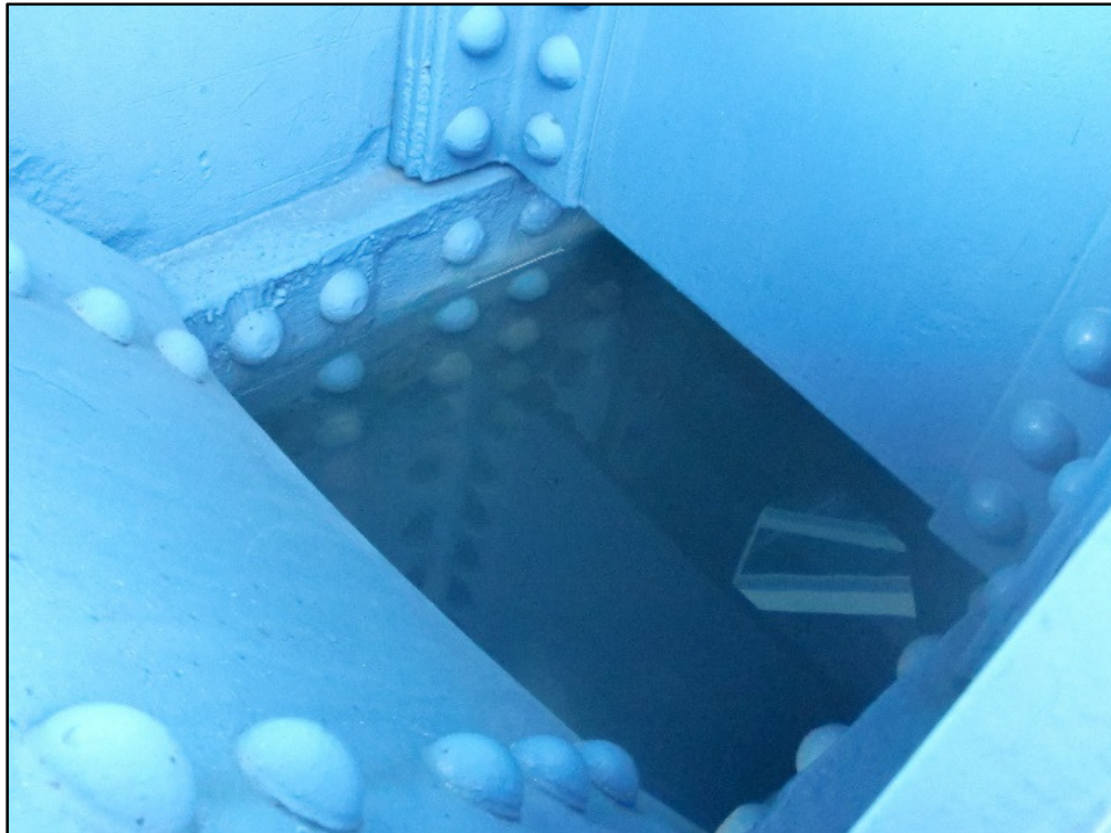
Photo 50 – Standing Water in Bearing Joint, Main Truss Spans.
