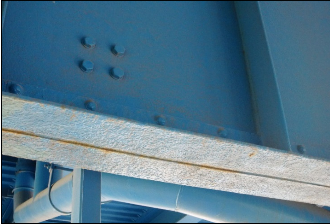
Photo 31 – Typical Floor Beam Bottom Flange Surface Pitting, Main Truss Spans.
