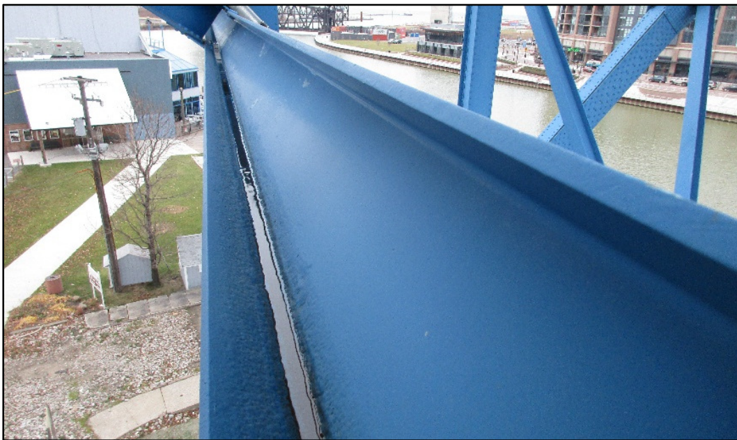
Photo 46 – Water Accumulation on Lower Lateral Bracing.
