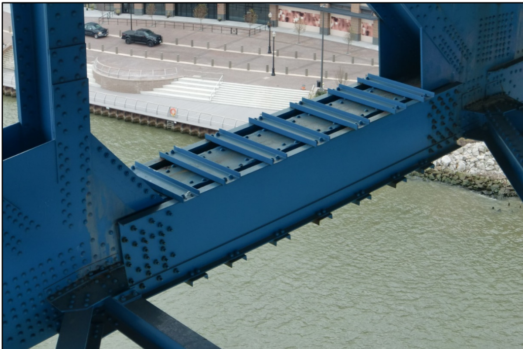
Photo 42 – 2007 Lower Chord Retrofit, L 24 L 25 , Span 8.
