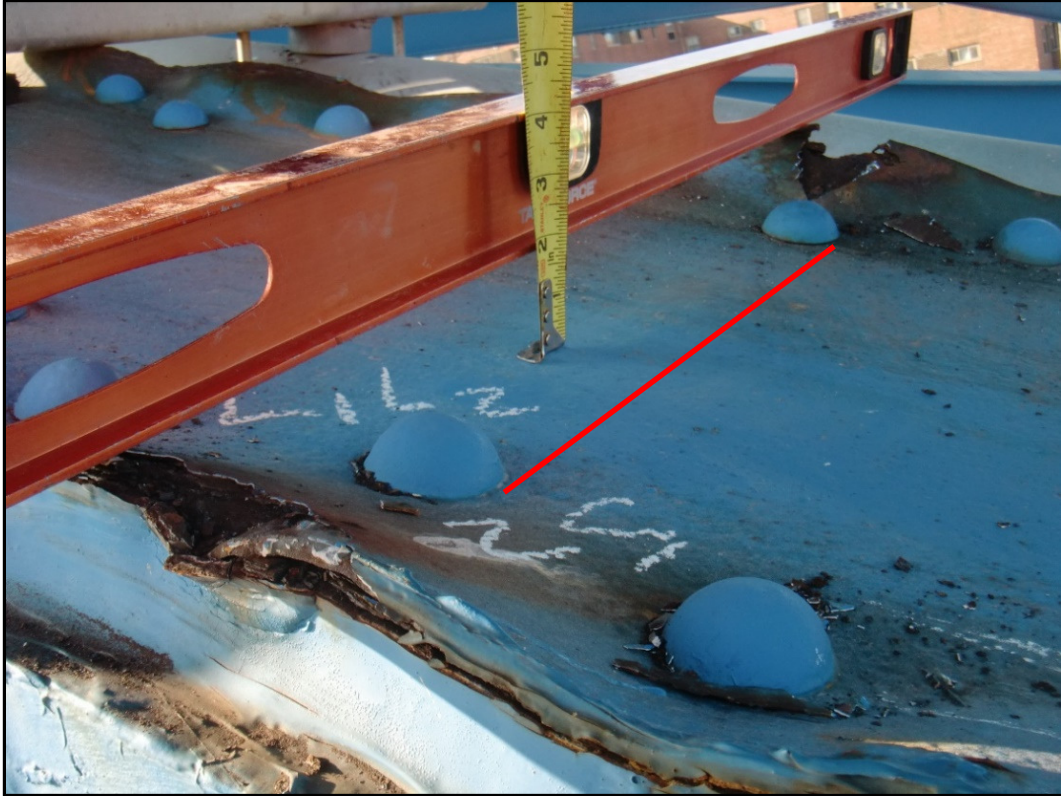
Photo 41 – Typical Lower Chord Plate Distortion Due to Pack Rust Distortion (Note: top plate is flat between inner rivets, shown by red line).
