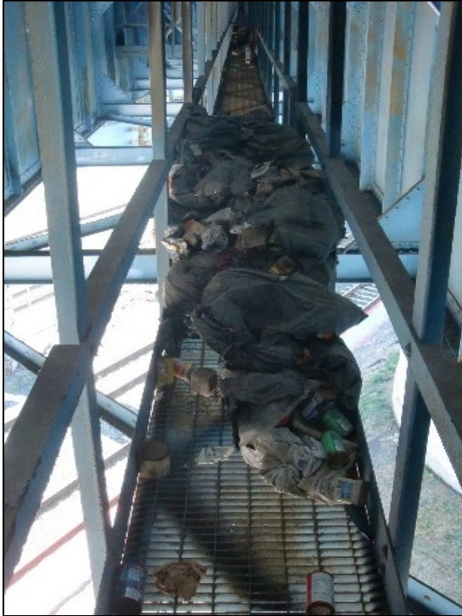
Photo 66 – Debris from Vagrants, Lakefront Ramp Catwalk.
