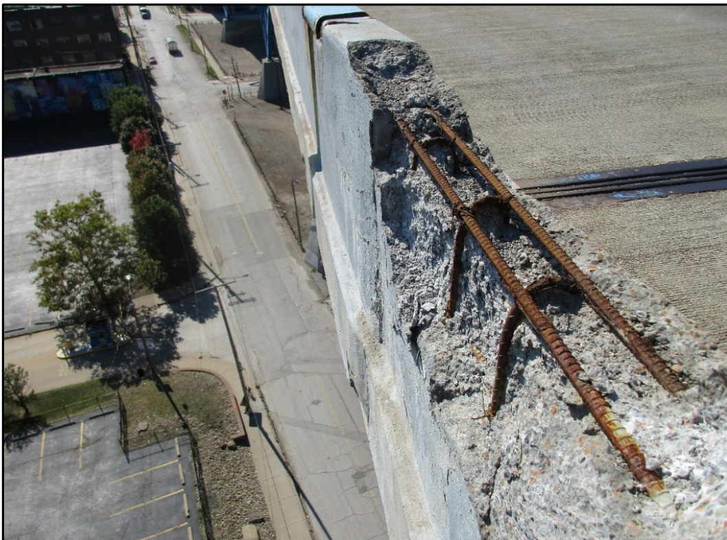
Photo 10 – Typical Top of Railing Spall, Span 7 South Railing.
