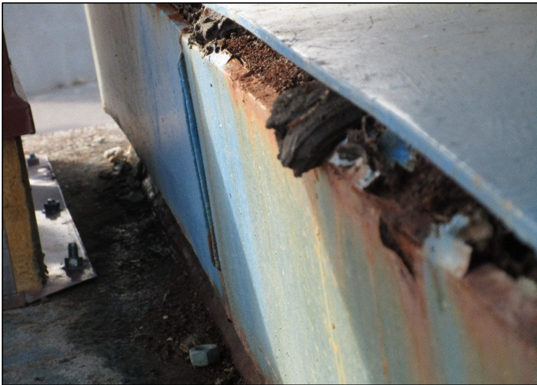
Photo 48 – Close-up of Debris & Steel Shot Blast within Expansion Bearing Box.
