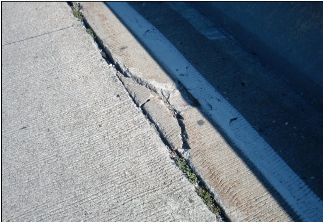
Photo 65 – Approach Slab Settlement, East Approach.
