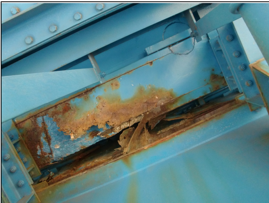
Photo 20 – Leakage through Damaged Joint Membrane, East Approach - Forward Section.
