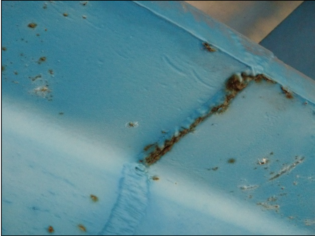
Photo 57 - Crevice between Adjacent Weld Passes, Girder GF2, Section C.
