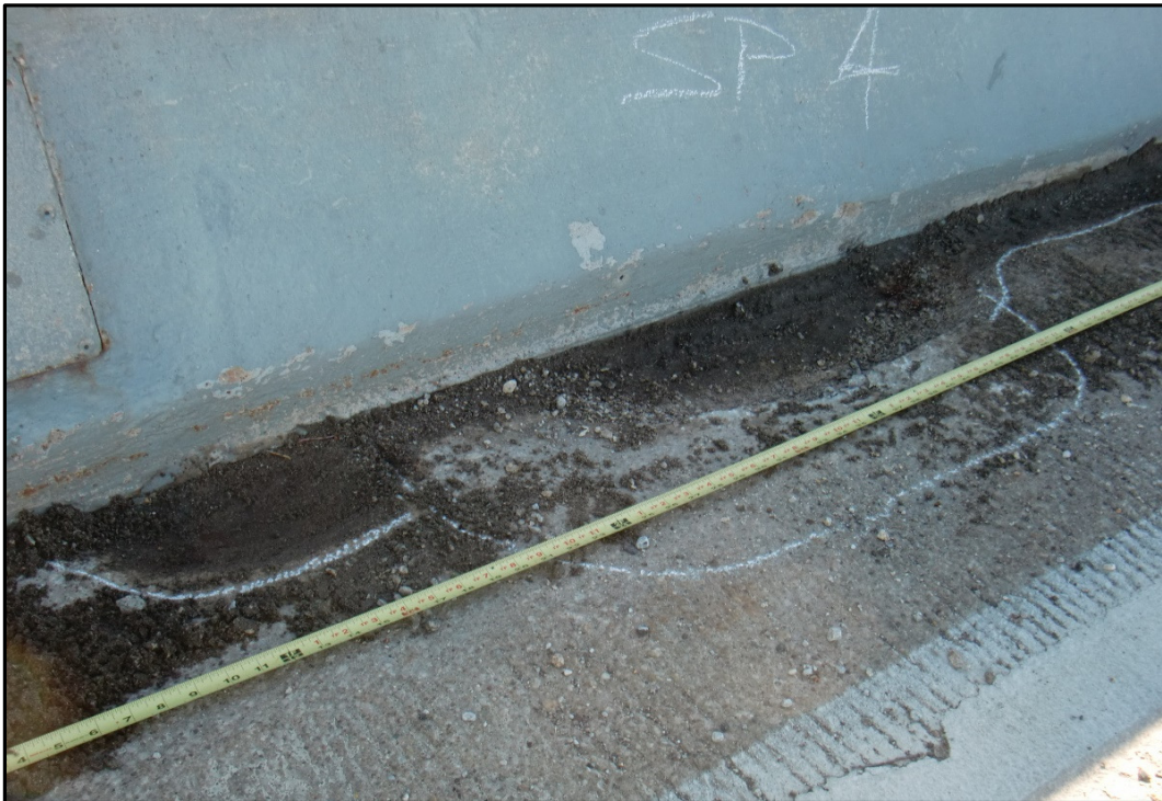
Photo 8 – Wearing Surface Spall Along Gutterline, Span 4.
