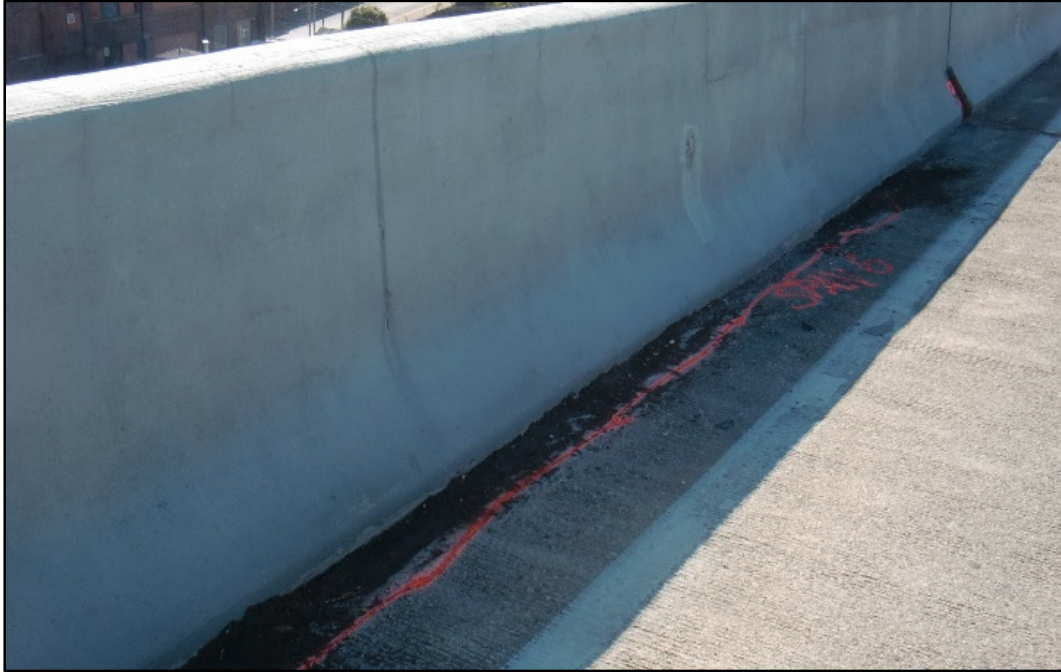
Photo 7 – Typical Gutterline Spalling, Wearing Surface.
