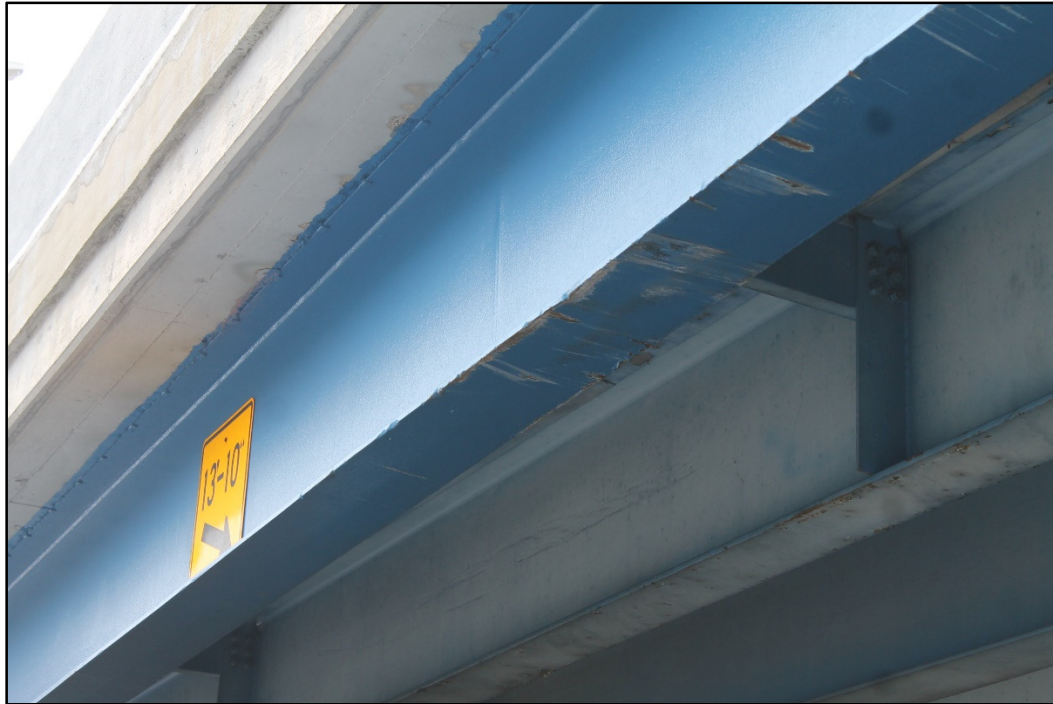
Photo 23 – Heat-Straightened & Repainted Beam FSS with New Vehicle Scrapes, over West 9 th Street.
