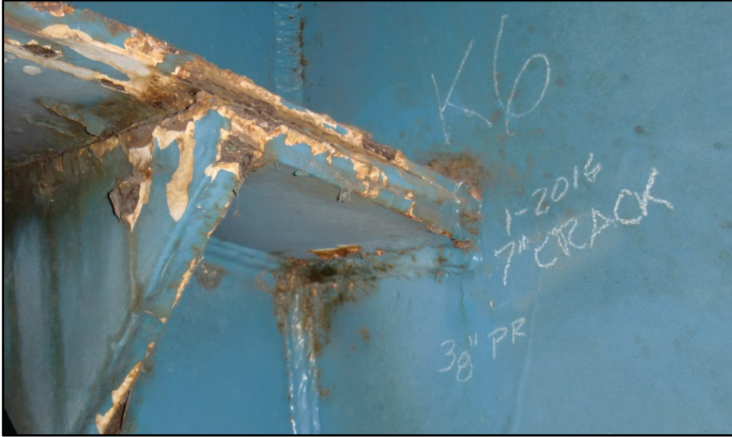
Photo 29 – New Pack Rust Induced Crack at Floor Beam Cantilever Seat at Column K6, Unit K (SR 2 EB over West 28 th Street).
