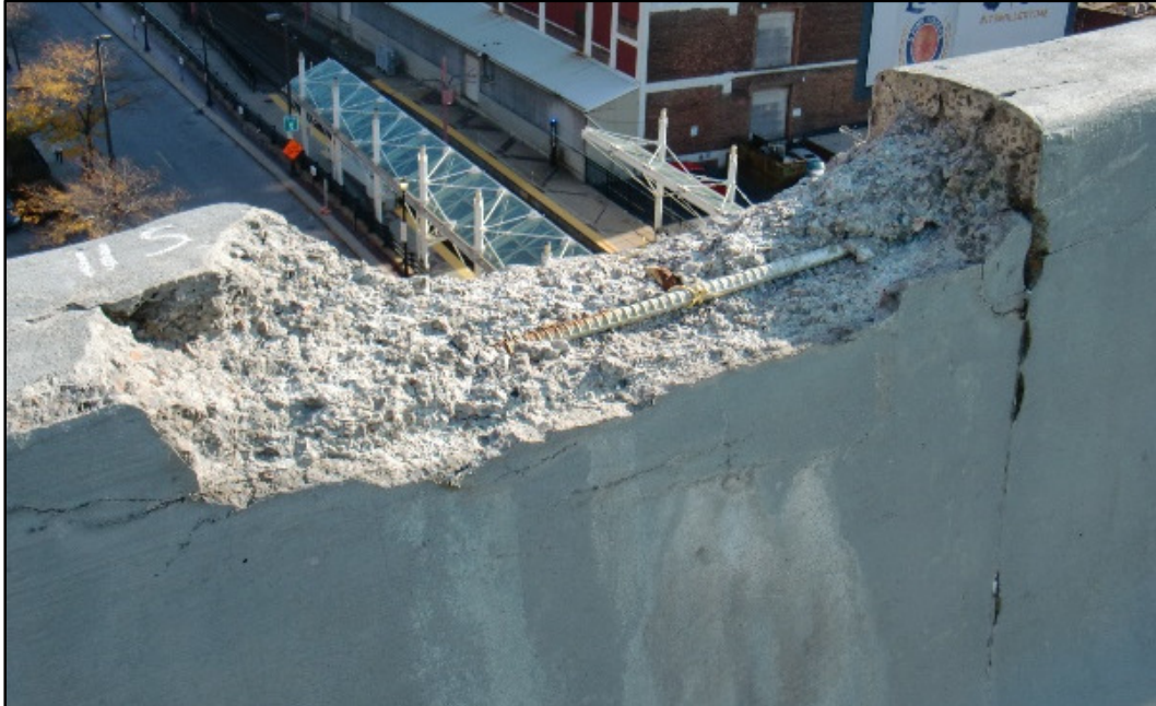
Photo 9 – Typical Top of Railing Spall without Corrosion, Span 7 South Railing.
