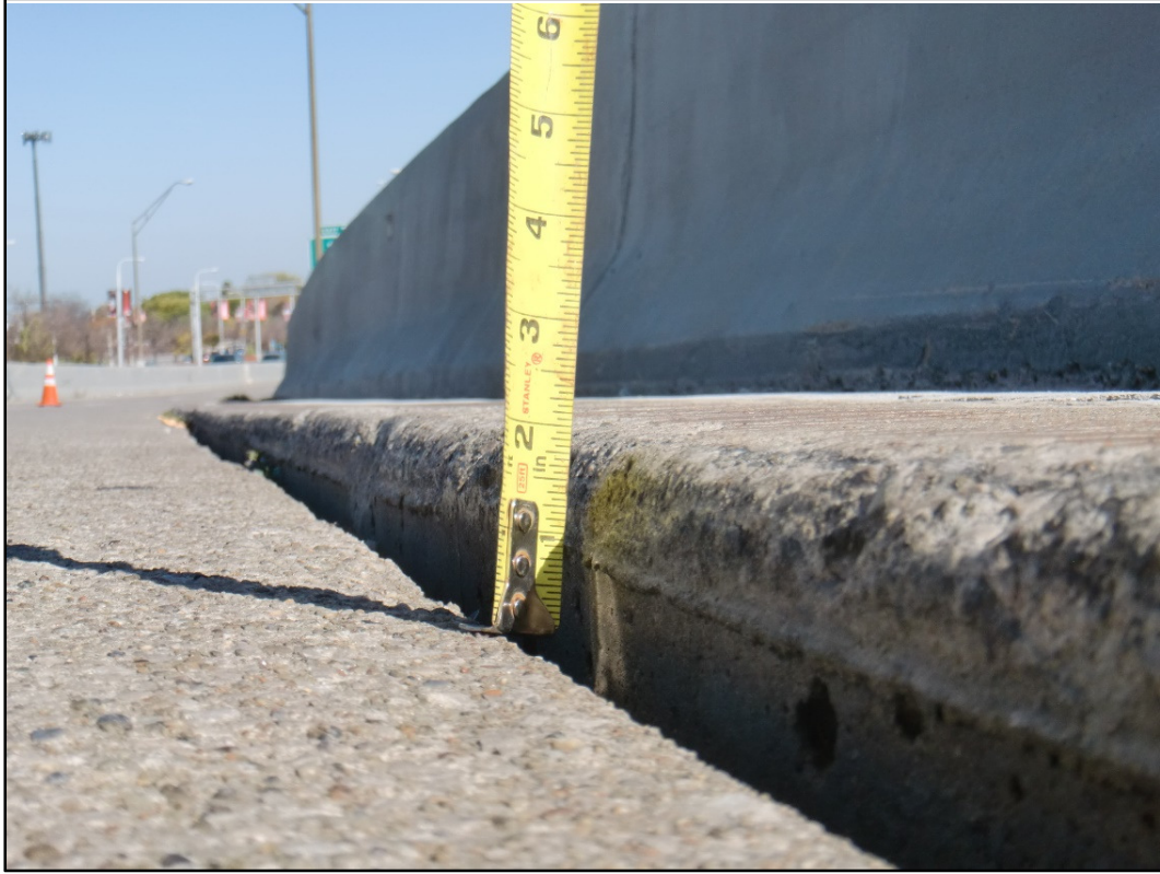
Photo 64 – Typical Condition, W 28 th St. Ramp.
