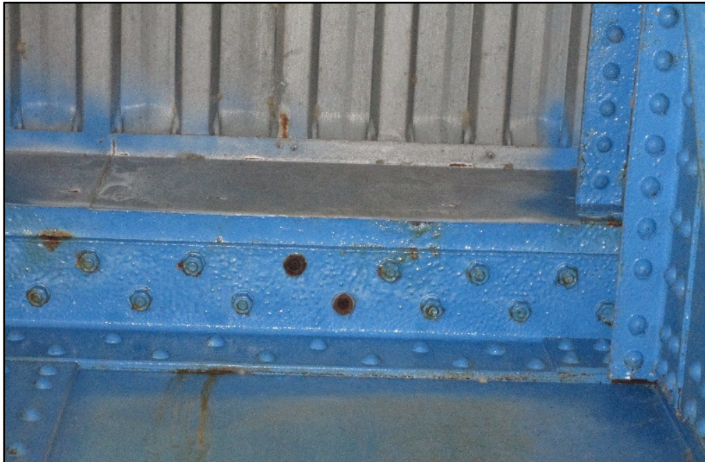
Photo 28 – Missing Bolts, Lakefront Ramp - East Approach.
