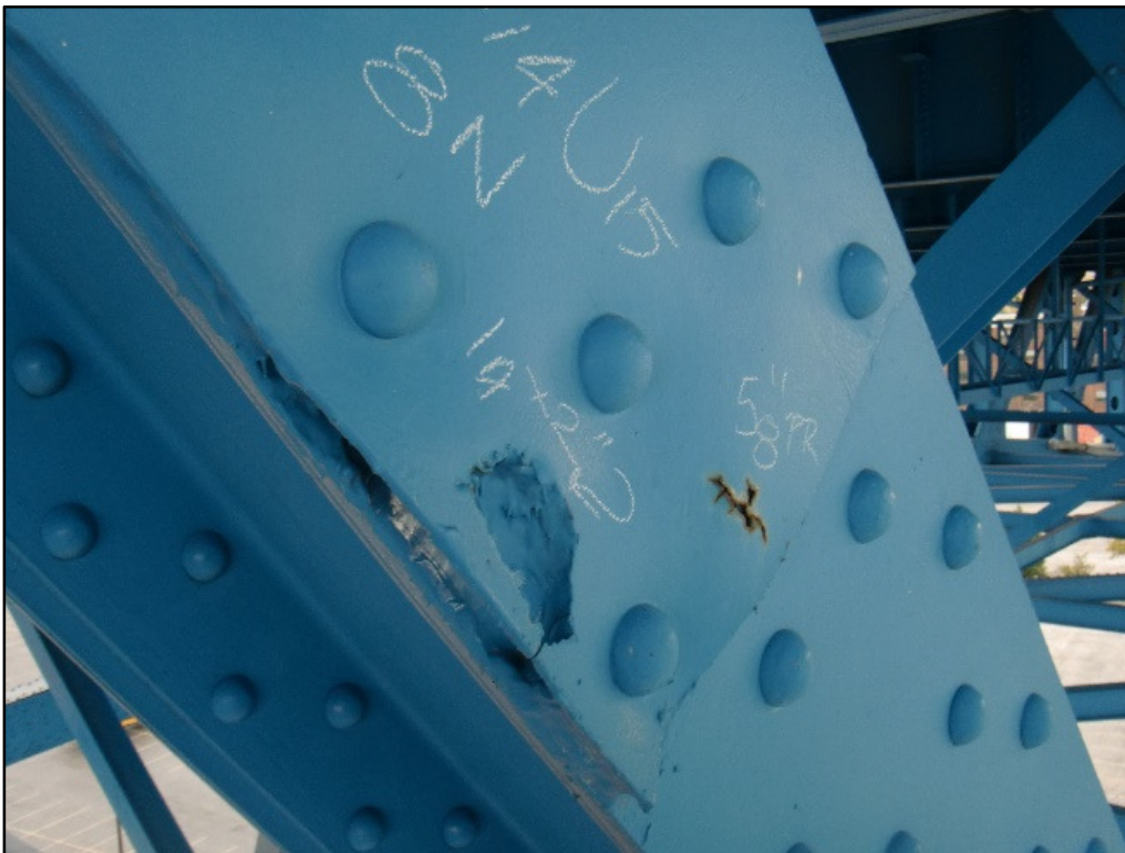
Photo 36 – \frac{5}{8} " Pack Rust Crack & Perforation in Fill Plate from Pack Rust, Diagonal U 14 U 15 , Span 8.
