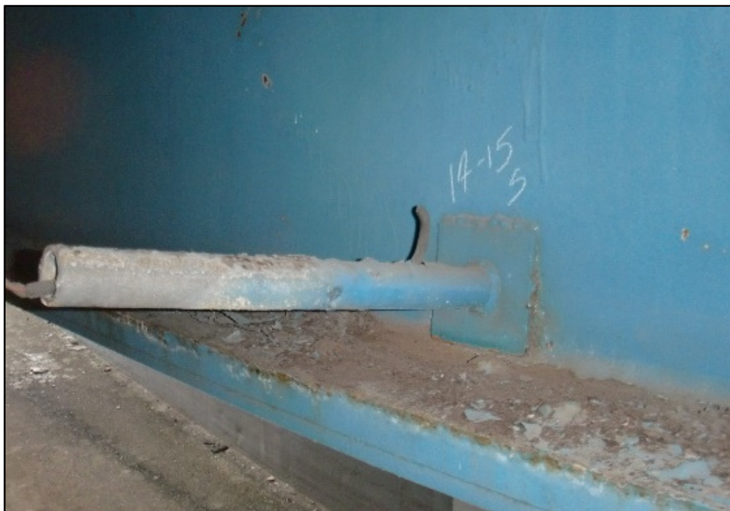
Photo 56 – Obsolete Utility Bracket Welded to South Twin Girder, Lakefront Trestle - East Approach.
