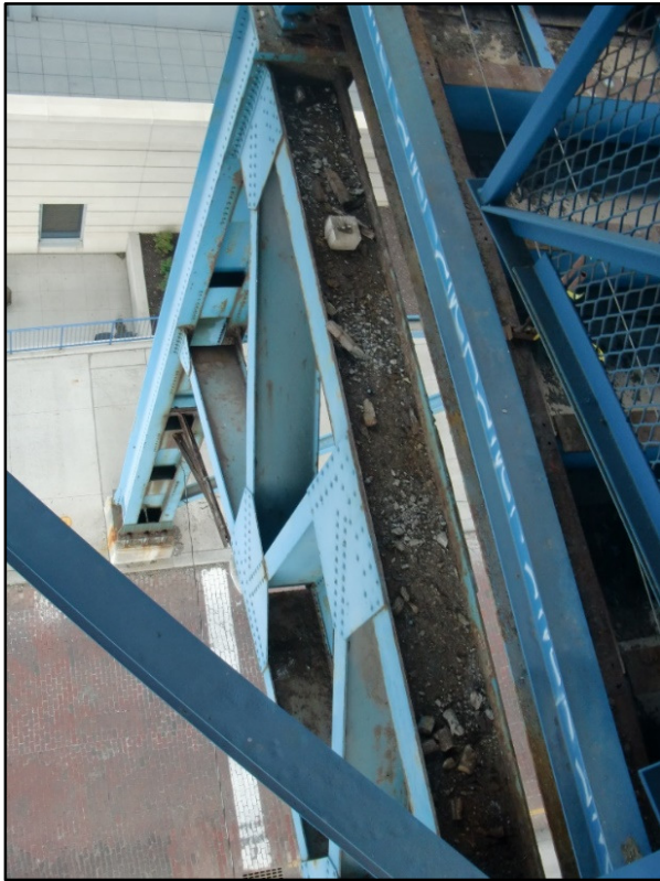
Photo 58 – Light Corrosion & Debris on Pier Bent 0/Pier 11.
