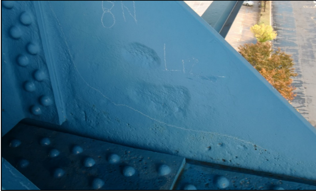
Photo 44 – Typical Gusset Plate Section Loss.
