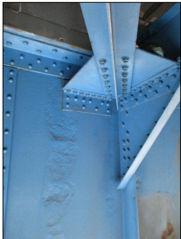
Photo 26 – Typical Surface Pitting, Lakefront Ramp - East Approach.
