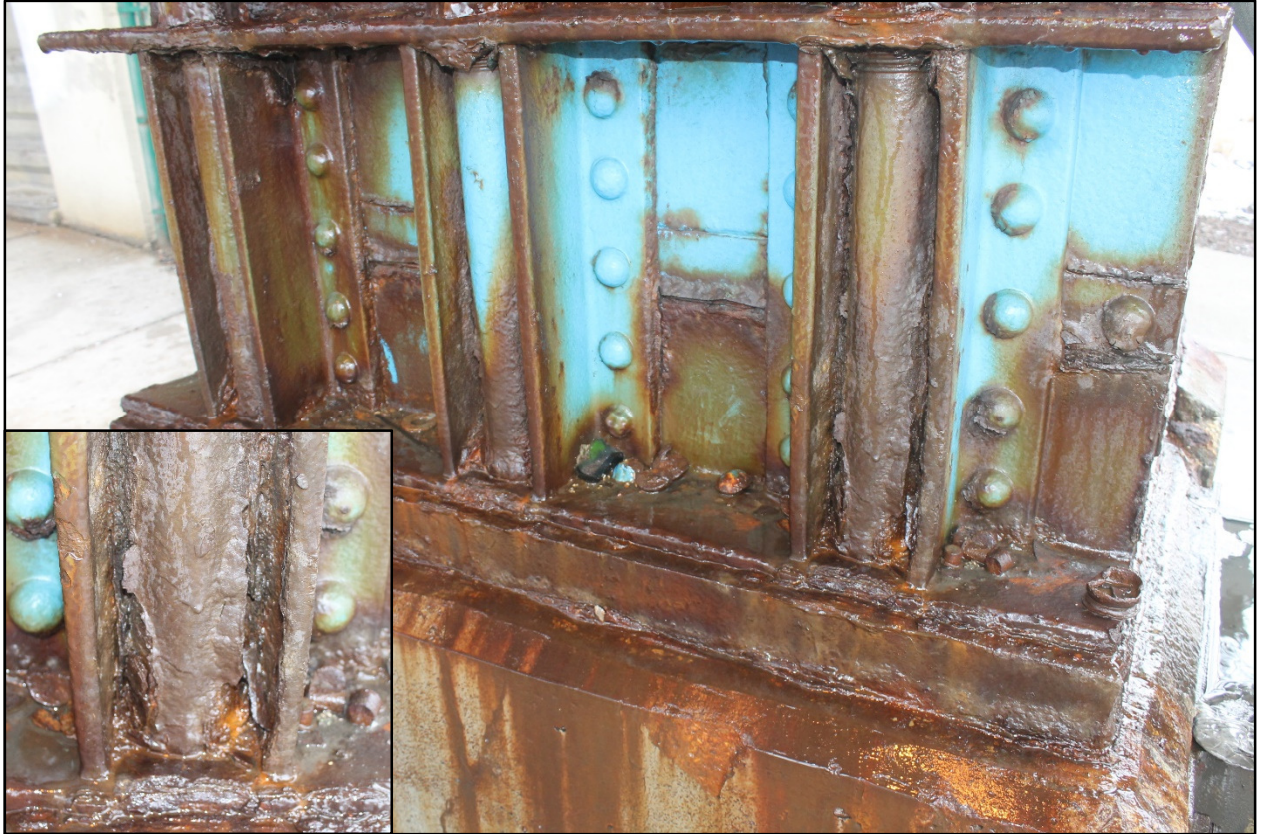
Photo 51 – Active Corrosion within Anchor Bolt Stiffener Chamber, Forward Approach.
