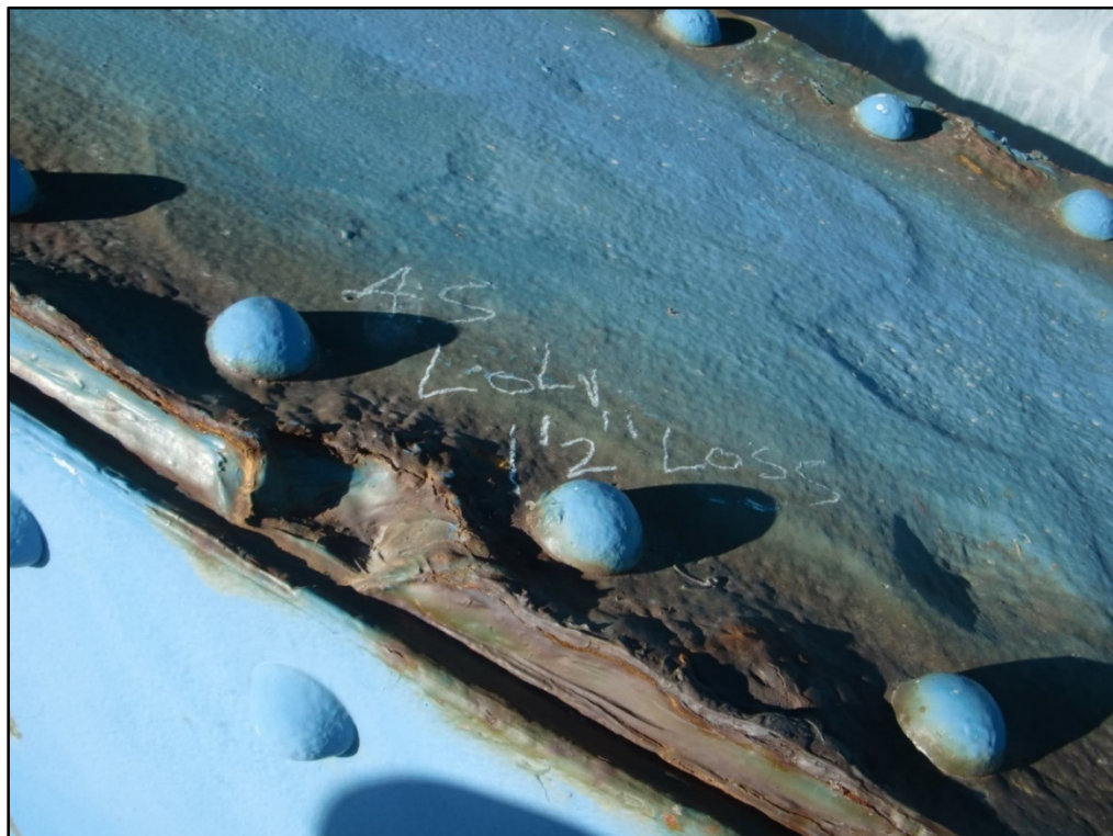
Photo 40 – Typical Lower Chord Pack Rust & Section Loss.
