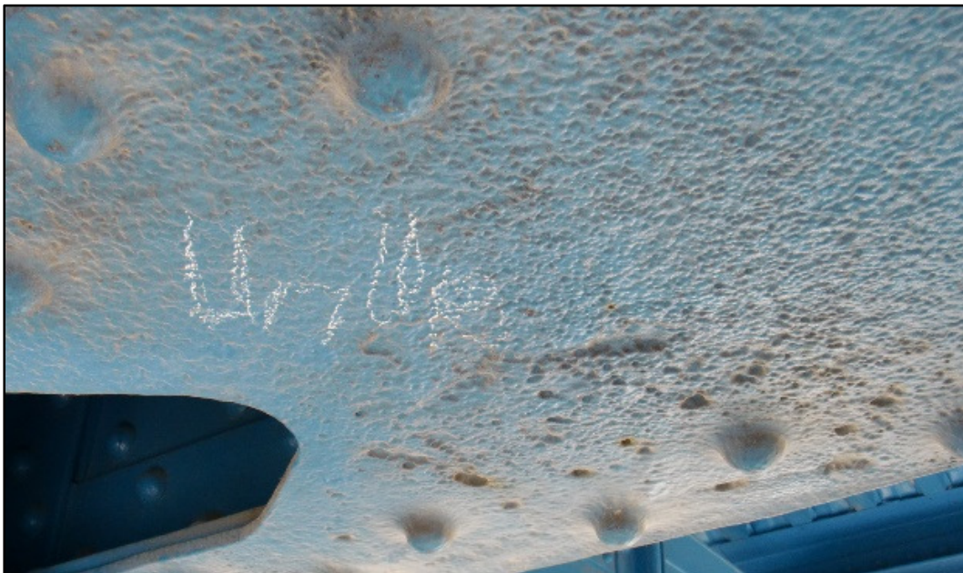
Photo 37 – Typical Surface Pitting, Main Truss Upper Chord.
