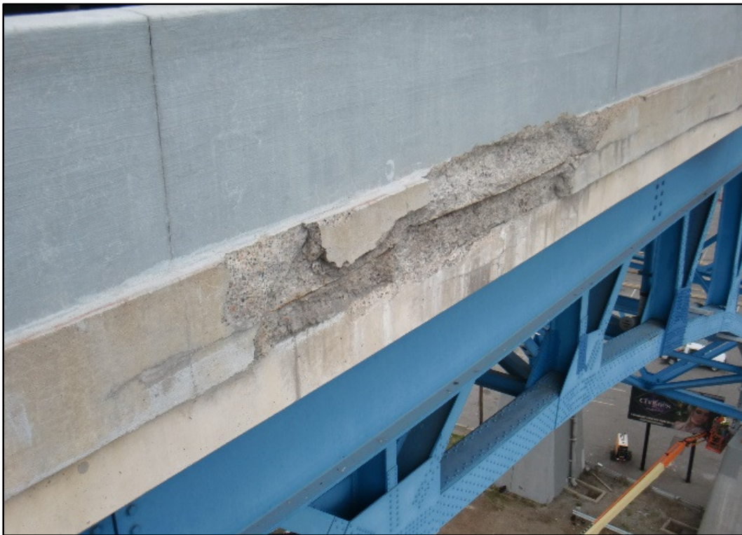
Photo 12 – Typical Spall and Delamination, Edge of Deck & Exterior Face of Parapet over Traffic.
