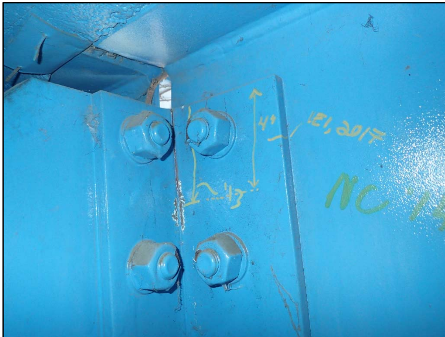
Photo 13 – Unit I, Section M, Floorbeam 2; 4" L vertical crack in south exterior stringer to floorbeam cantilever connection angle
