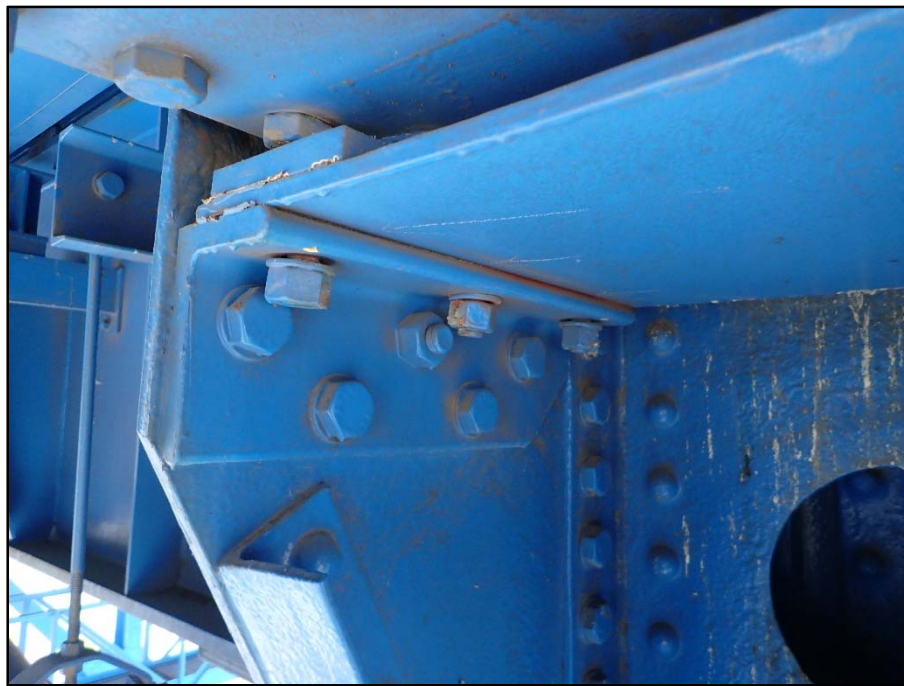
Photo 30 – Span 4, Floorbeam 0; Loose bolts on the inboard sliding plate for the north truss at U0
