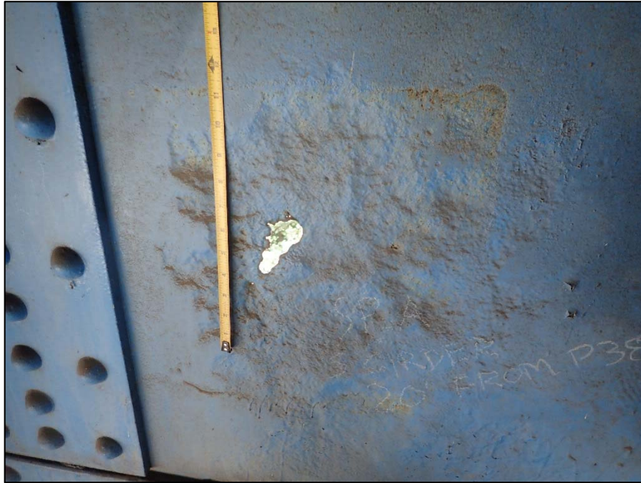
Photo 26 – Unit V, Span 38, South girder, north face; 3" H x 1" L corrosion hole 2' above bottom flange
