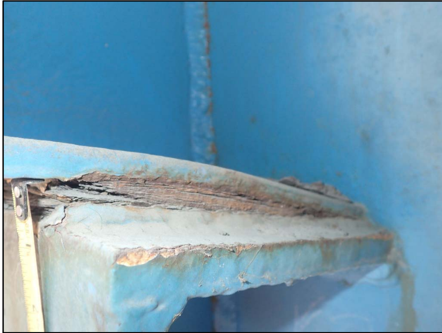
Photo 12 – Unit I, Section K, Floorbeam 2; 6" Long horizontal crack
