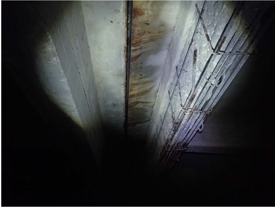
Photo 1 – Unit I, Joint T1; Leaking joint resulting in corrosion staining and efflorescence
