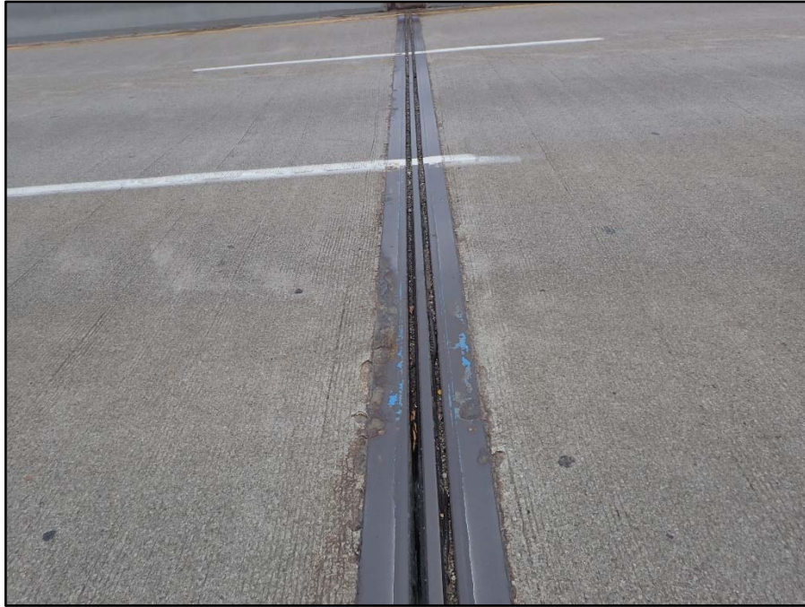
Photo 3 – Unit II, Joint L; Failed joint seal
