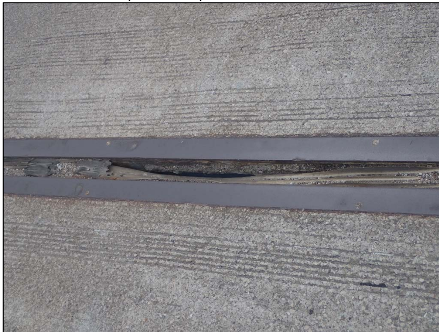
Photo 10 – Unit IV, Joint A; 4' L section of joint has failed along middle
