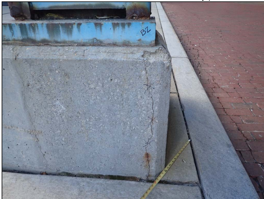
Photo 42 – Unit III, Framed and Braced Column; Bent 2, north column; Full Height x 1/16" W vertical crack on the southwest corner
