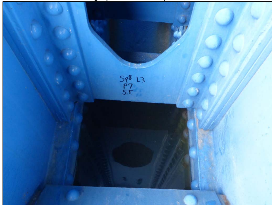
Photo 33 – Span 2, South truss, L2L3; Panel point L3 is full of water
