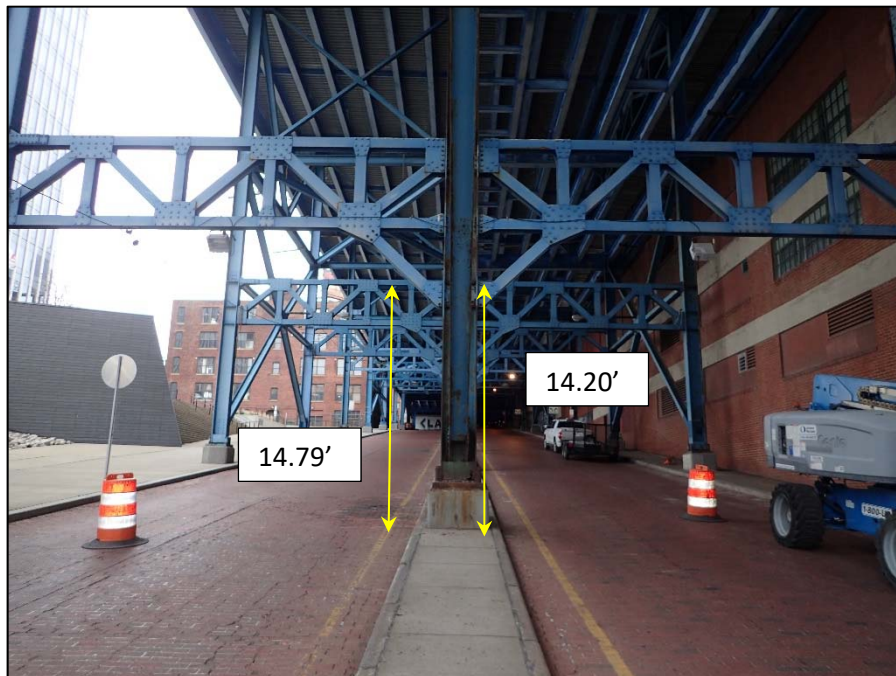
Unit III, Frame & Braced Column Section; Main Avenue, Looking East below Trestle
