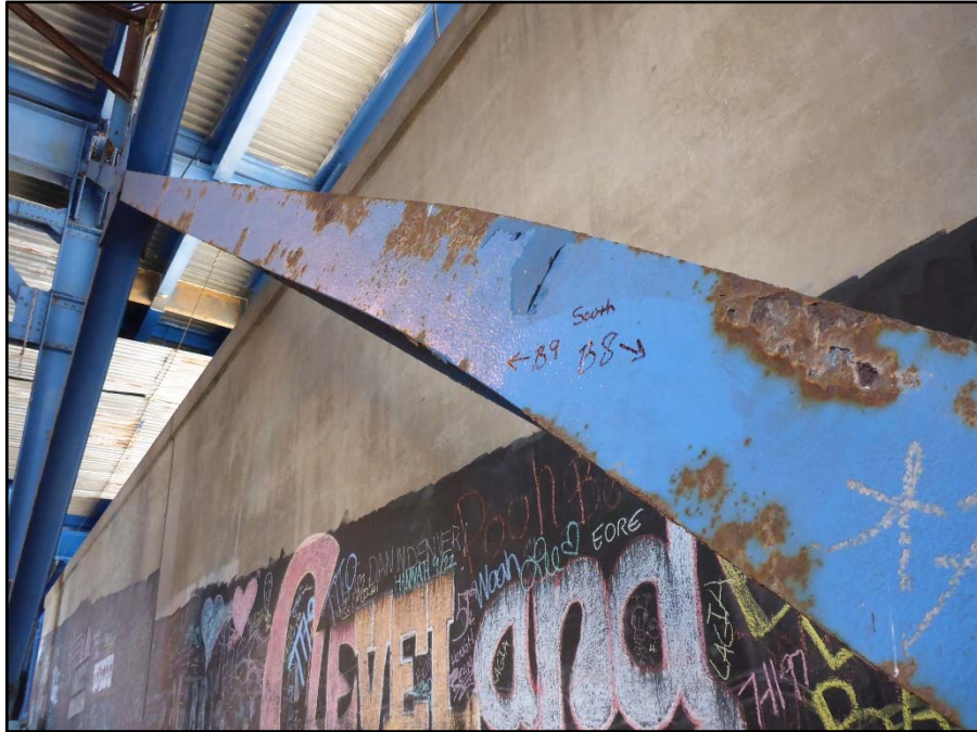
Photo 22 – Unit III, Bent 8-9, South column; Diagonal from Bent 8 to Bent 9 is bent upward and to the South due to collision damage
