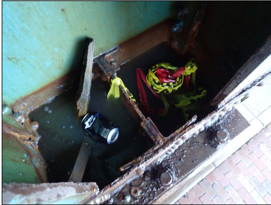
Photo 39 – Unit III, Bent 11, South column; Base of column is holding water
