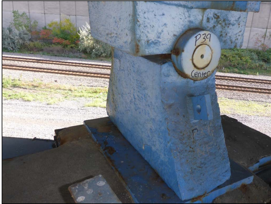
Photo 28 – Unit V, Span 40, center bearing; 1/8" D painted over pitting
