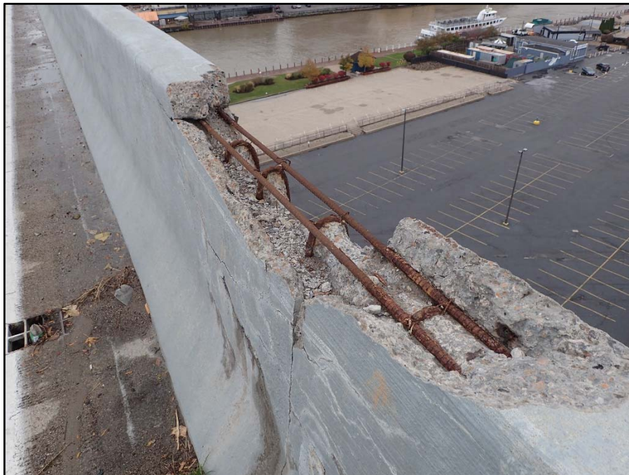
Photo 4 – Unit II, Joint K, bridge parapet; 6' L x Full Width x 18" H spall
