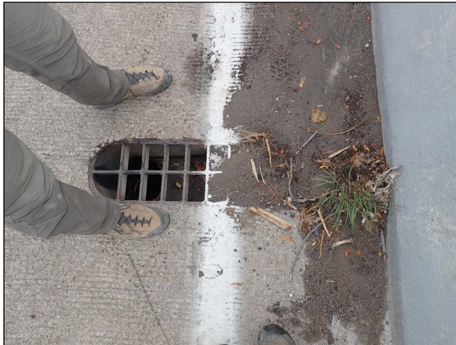
Photo 2 – Unit II, Joint L1; 3/4 blocked curb drain
