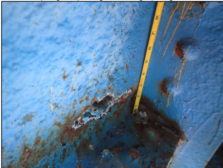
Photo 21 – Unit III, Bent 4, North column; 5-1/2" W x 1/2" H corrosion hole above bearing plate
