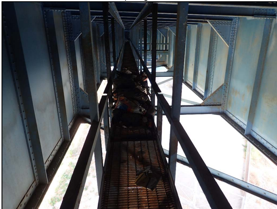
Photo 29 – Unit V, Span 41; Debris and trash on the catwalk
