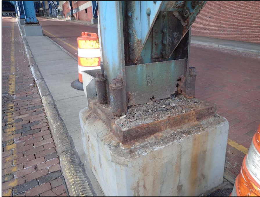
Photo 41 – Unit III, Framed and Braced Column; Bent 1, middle column; 8" H x 6" W corrosion hole in the stay plates
