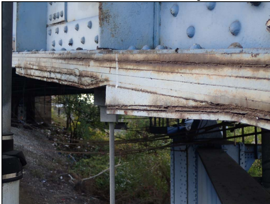
Photo 27 – Unit V, Spans 38 – 39, South Girder; Up to 1-1/4" T pack rust between bottom flange plates
