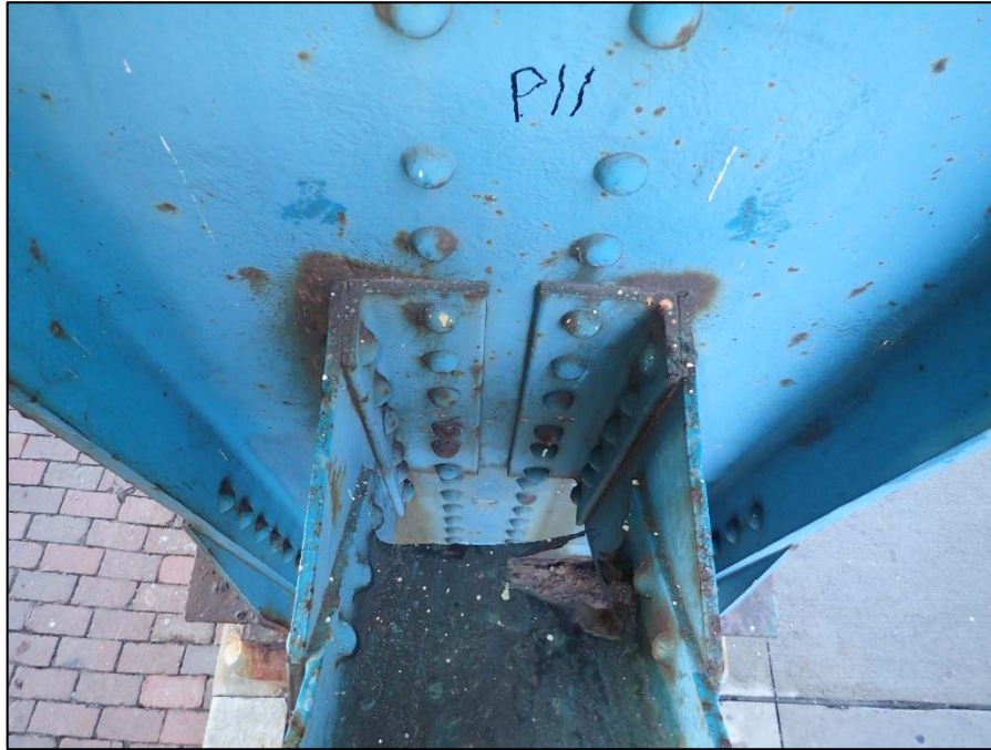
Photo 18 – Unit III, Span 11, North column; 1/4" T pack rust at connection and 4" Diameter corrosion hole through web of brace
