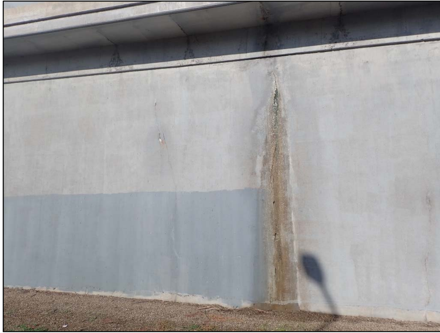
Photo 47 – Unit V, East abutment, South wingwall; Full Height vertical cracking with moisture staining and efflorescence spaced 10'-15' apart
