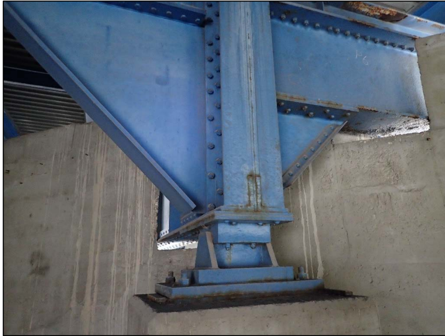
Photo 16 – Unit I, Section N, Floorbeam 7, center bearing; Typical bearing paint condition
