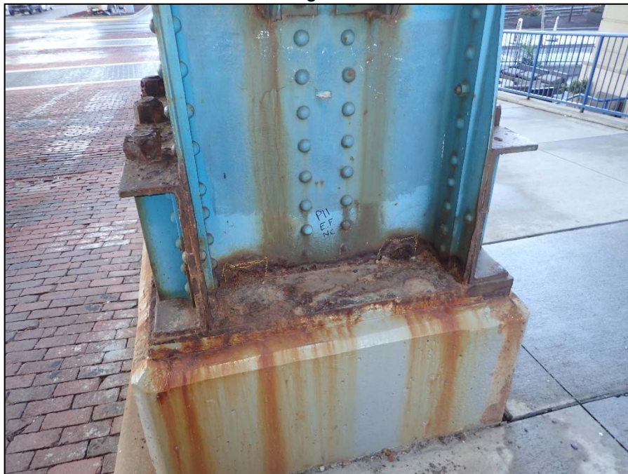
Photo 40 – Unit III, Bent 11, North column; Plugged drain holes and up to 10% section loss along anchor bolts
