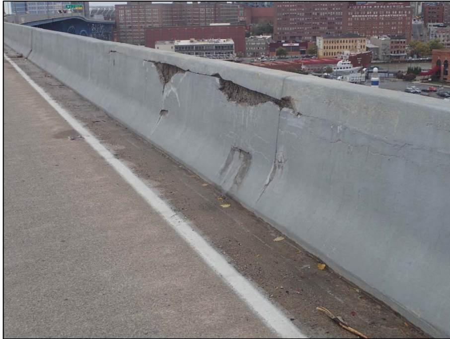
Photo 5 – Unit III, South parapet at 30+50; 15' L x 15" H x up to 4" D with exposed rebar
