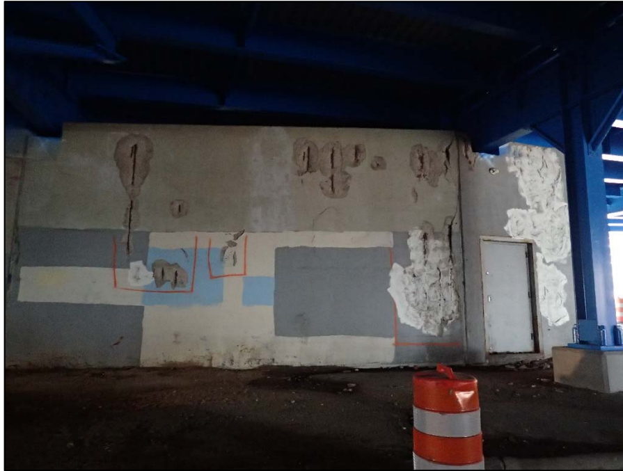
Photo 45 – Unit IV; West Lakeside entrance ramp; West face of south wall exhibits multiple spalls with exposed reinforcement
