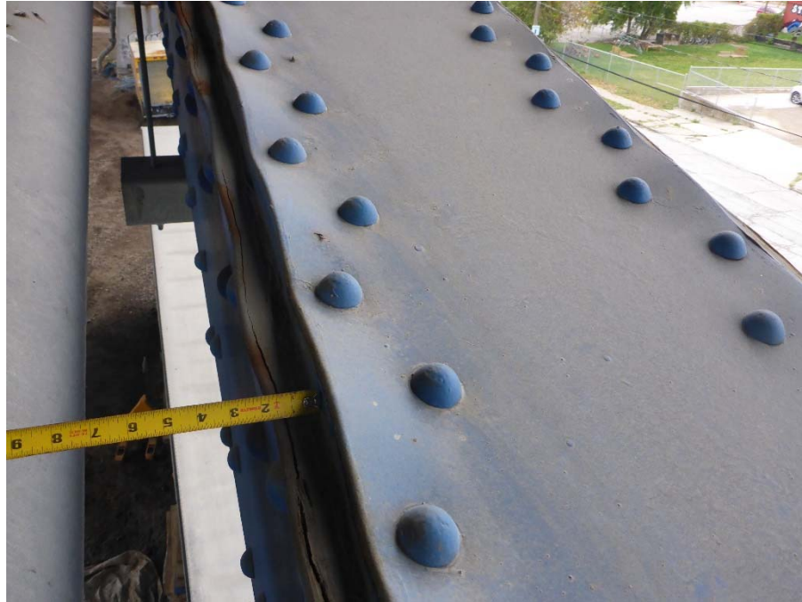
Photo 32 – Span 1, South truss, L2L3; 1" T pack rust distorting top flange plate and web plates
