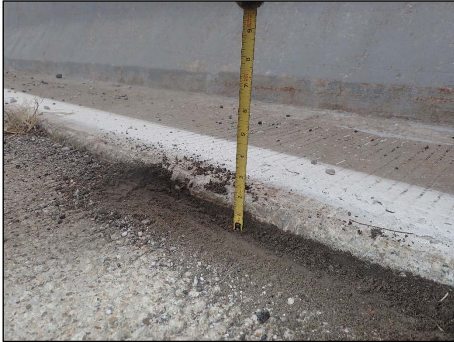
Photo 11 – Unit V, Westbound lanes; East Approach roadway; North "curb" height varies 1-2" above the roadway
