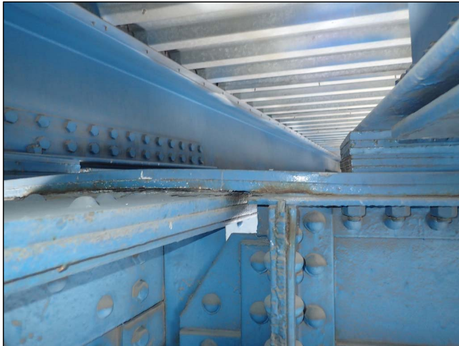
Photo 15 – Unit I, Section N Girder 5; 1/2" T pack rust between girder top flange and cantilever support tie plate
