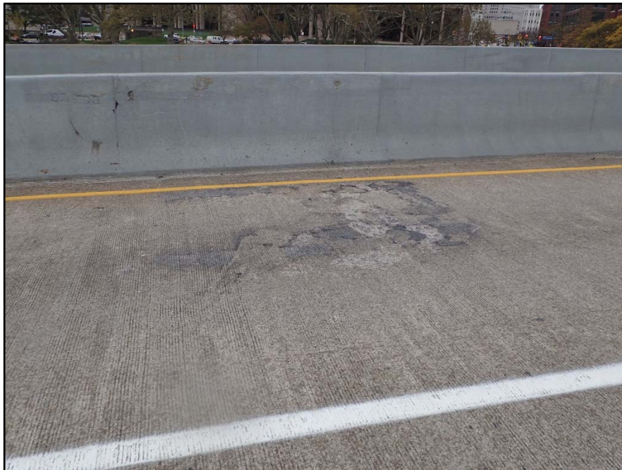
Photo 8 – Unit IV; Westbound lanes, South Lane; 8' L x 8' W area of 1" D spalling with staining
