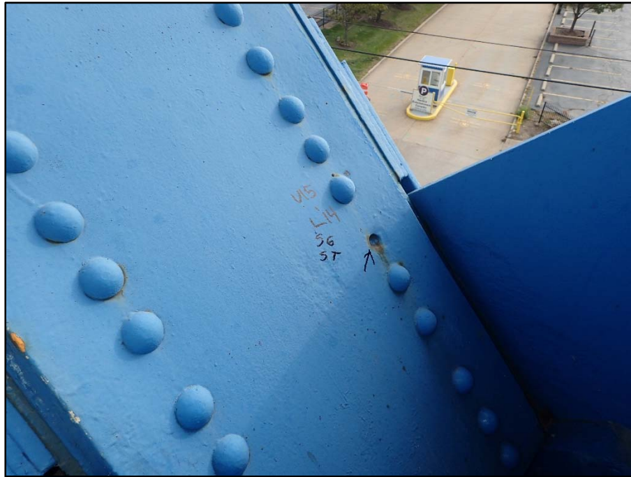
Photo 34 – Span 6, South truss, L14L15; Popped rivet head at L14
