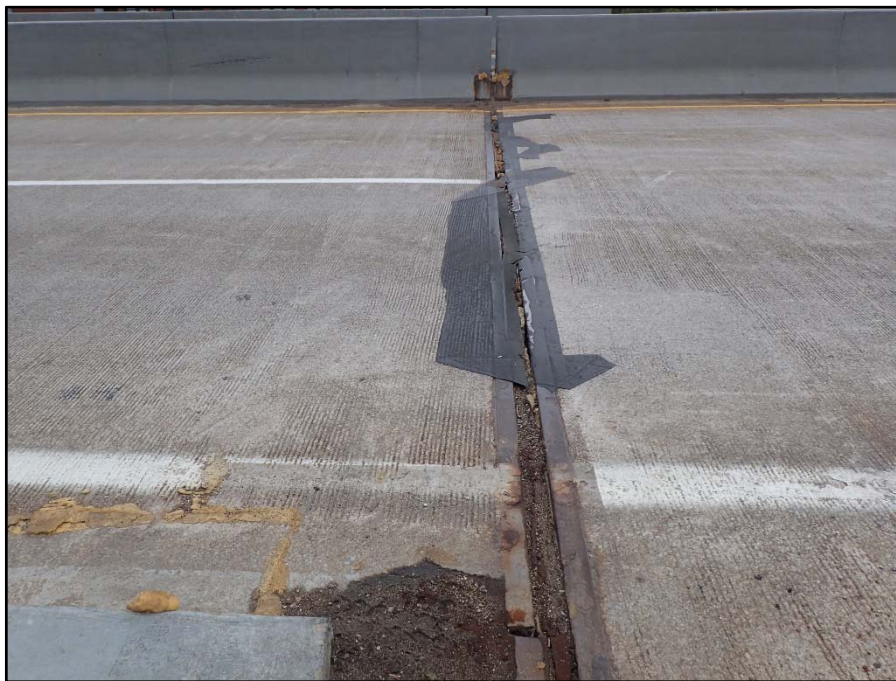
Photo 6 – Unit IV; Entrance Ramp, Westbound lanes; Failed joint
