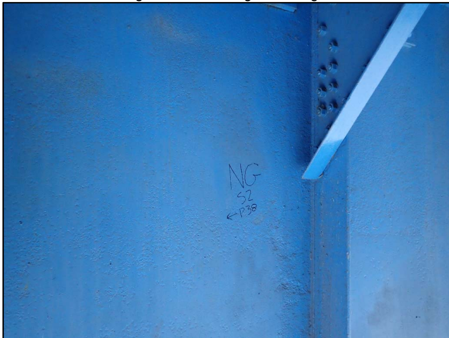
Photo 25 – Unit V, Typical girder; Up to 1/16" D painted over pitting
