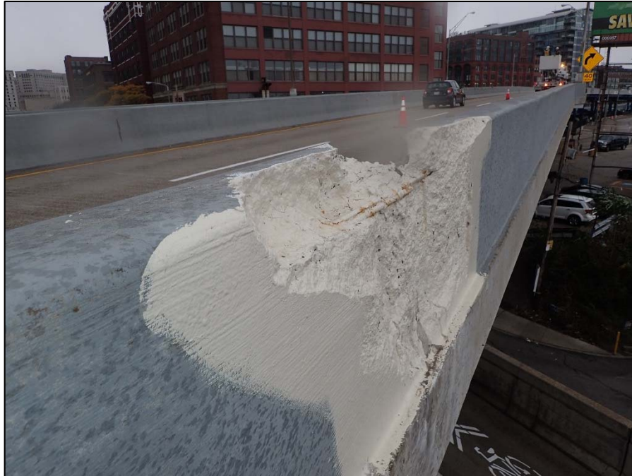
Photo 9 – Unit IV, Section H, Westbound lane; 6' L x Full Width x 6" D spall with exposed reinforcement
