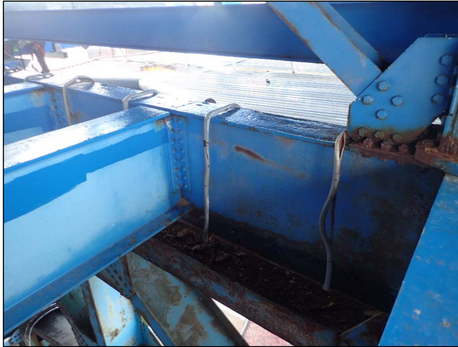
Photo 20 – Unit III, Bent 0 floorbeam; Typical 3/16" D painted over pitting with ponding water along top flanges
