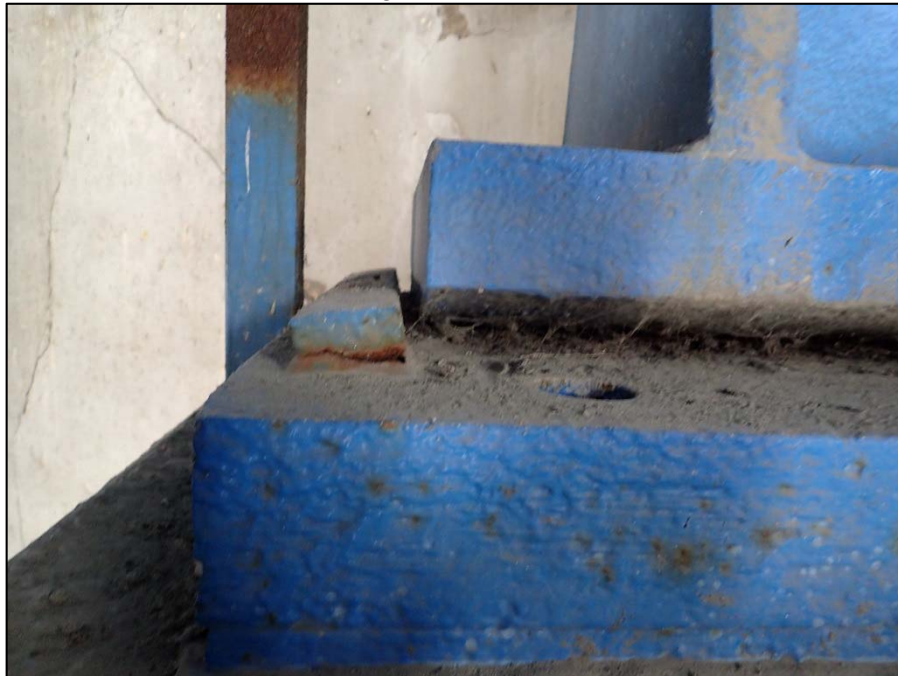
Photo 17 – Unit I, Section N at Floorbeam 8, North girder; South guide bar welds are cracked
