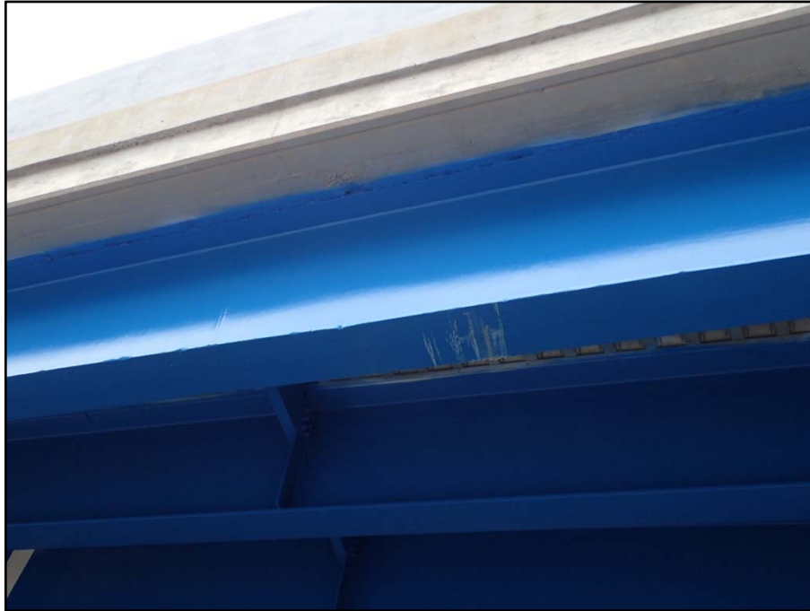
Photo 24 – Unit III, Bent 11 – 12; Over height vehicle collision damage to bottom flange of Stringer 1
