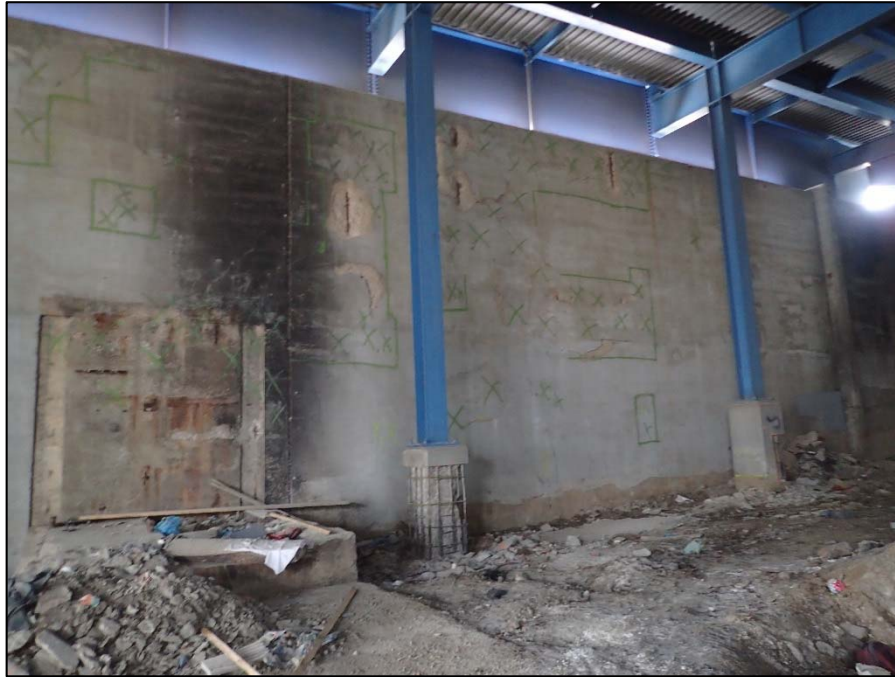
Photo 37 – Unit I, Section N; Southeast curtainwall is mapped out with areas of delaminations and spall to be repaired
