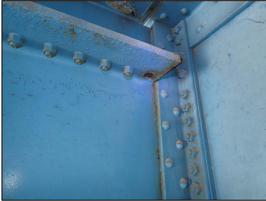
Photo 14 – Unit I, Section N; Popped rivet at end of top flange due to pack rust
