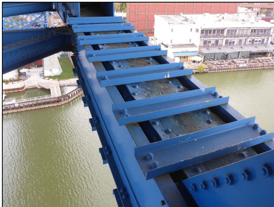
Photo 35 – Span 8, South truss, L24L25; Lower chord retrofit
