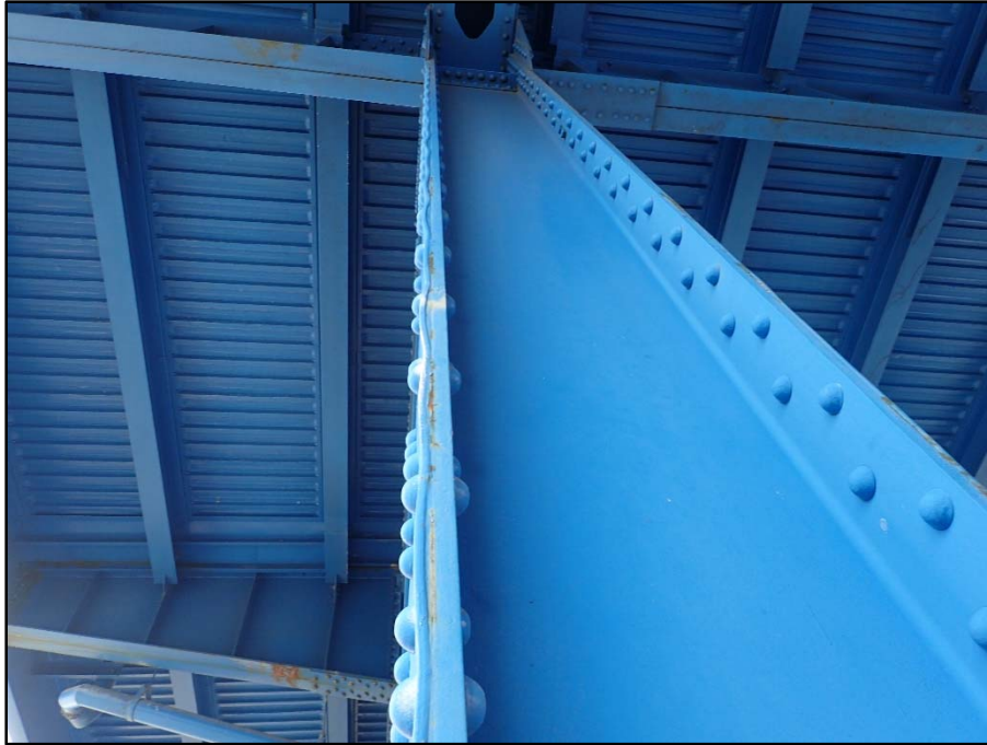
Photo 31 – Span 2, North Truss, L15U15; 3/4" T reactivating pack rust and scalloping of edges
