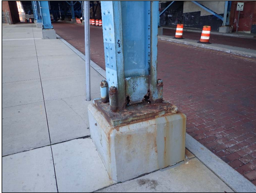
Photo 43 – Unit III, Framed and Braced column; North column exhibits 1/16" D pitting along the base
