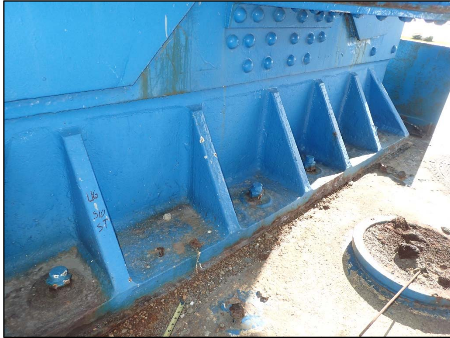
Photo 36 – Span 10, South Truss, L6 bearing; Anchor bolts nuts exhibit up to 50% section loss
