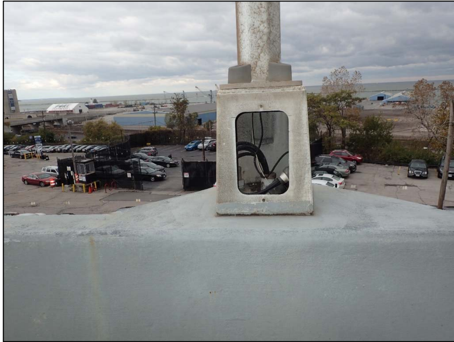
Photo 7 – Unit IV, Section E, North parapet; Missing light base cover
