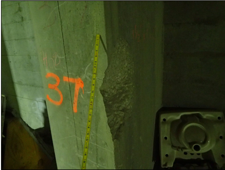
Photo 11 – Unit I, Section D, Frame 37; North column with 1'-10" H x 1' W x 3" D spall
