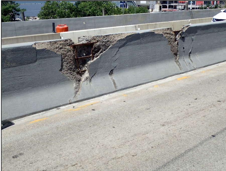
Photo 3 – Unit IV, Section E; Spalling along full height of median, South face
