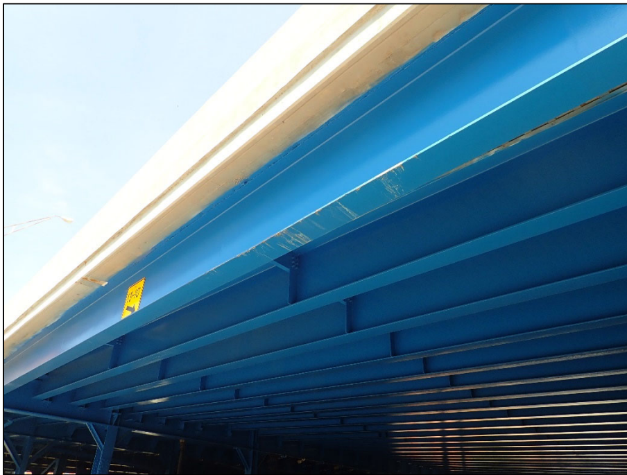
Photo 10 – Unit III, Bent 11/12; Stringer 1 with chipped paint on bottom flange over 9 th Street
