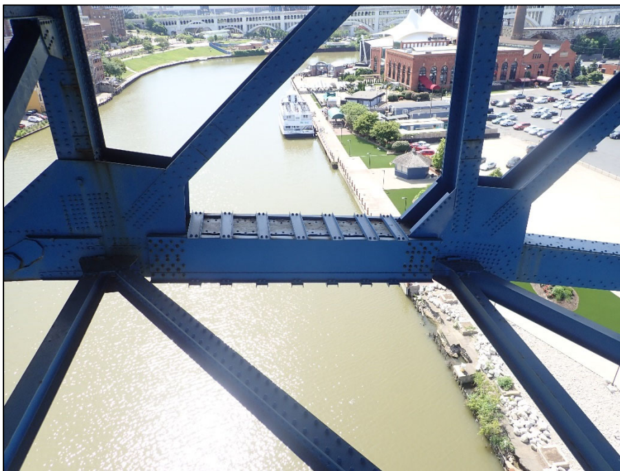
Photo 40 - Unit II, Span 8, South truss, L24L25; lower chord steel channel retrofit
