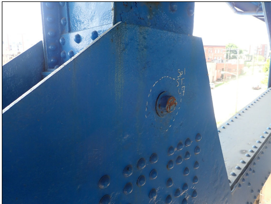
Photo 44 – Unit II, Span 1, South truss at L7; 3/16" D painted over pitting inboard gusset plate
