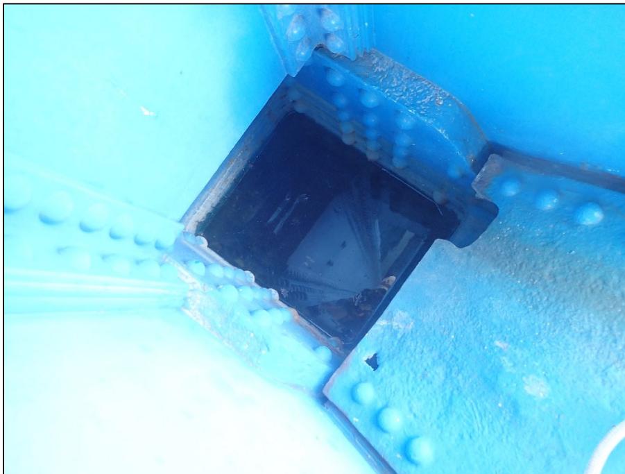
Photo 34 – Unit II, Span 4, South truss at L2; Bearing full of water, 3-1/2" L x 4" W corrosion hole in top plate
