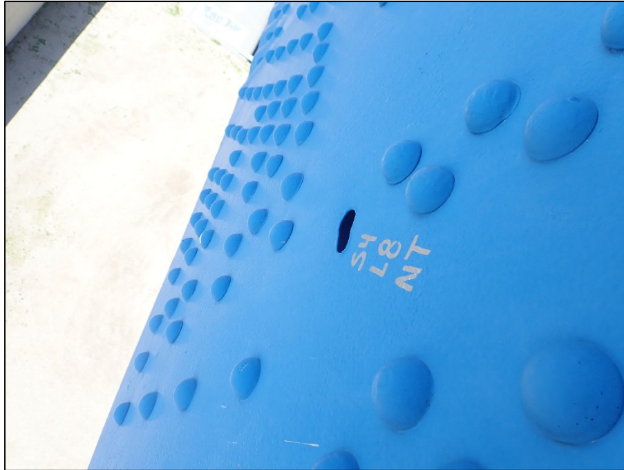
Photo 45 – Unit II, Span 4, North truss at L8; 2" Diameter corrosion hole in outboard gusset plate
