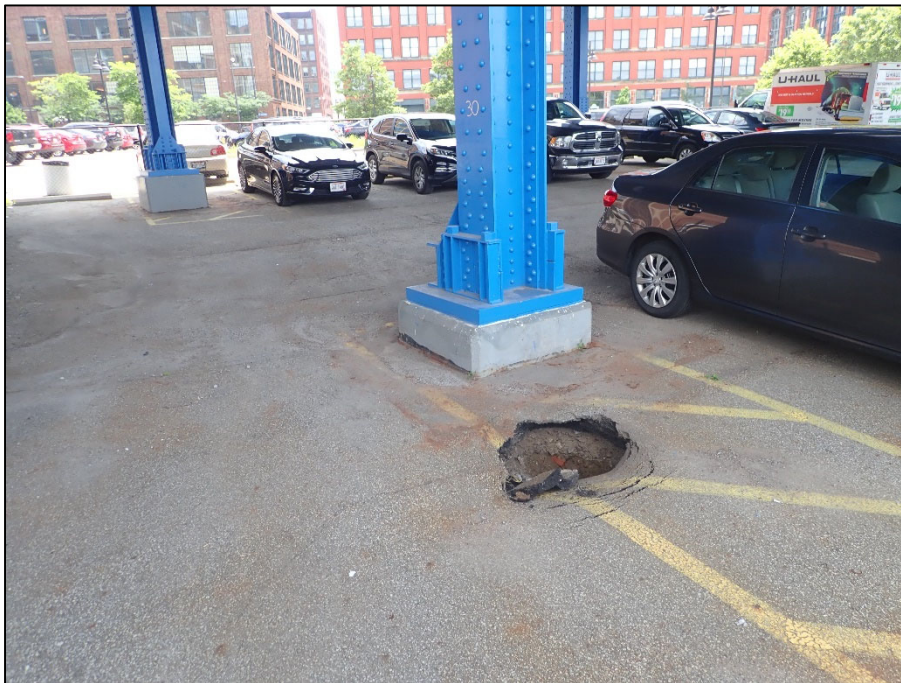
Photo 14 – Unit IV, Bent 30; 3' Diameter x 3' D sink hole near North column
