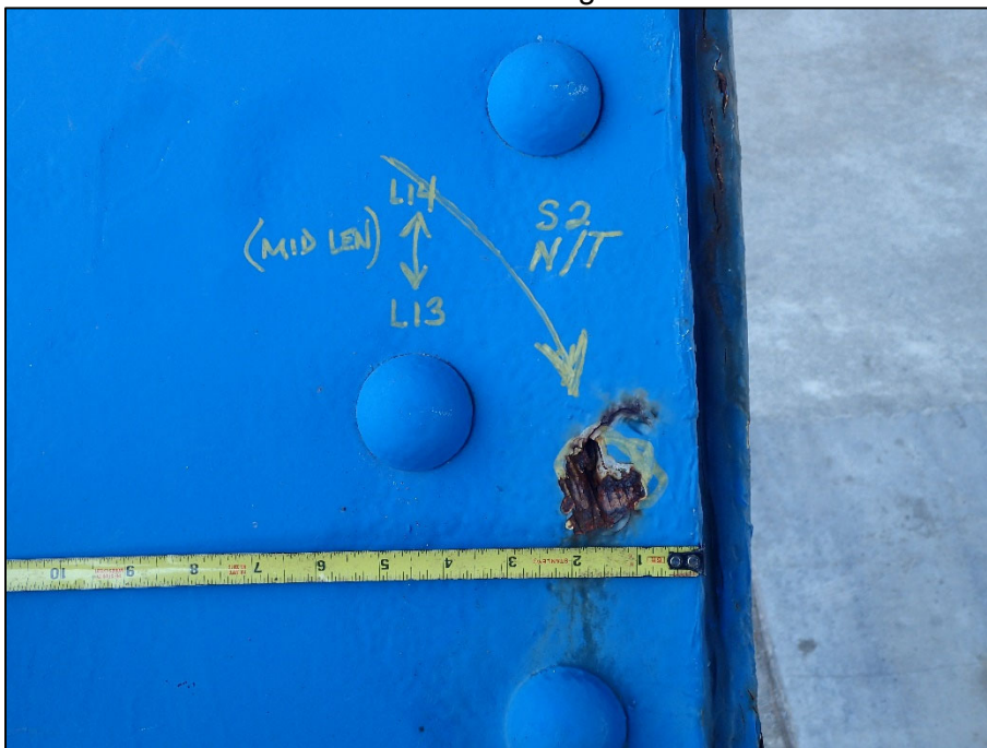
Photo 26 – Unit II, Span 2, North truss, L13L14; 1" Diameter corrosion hole in top plate
