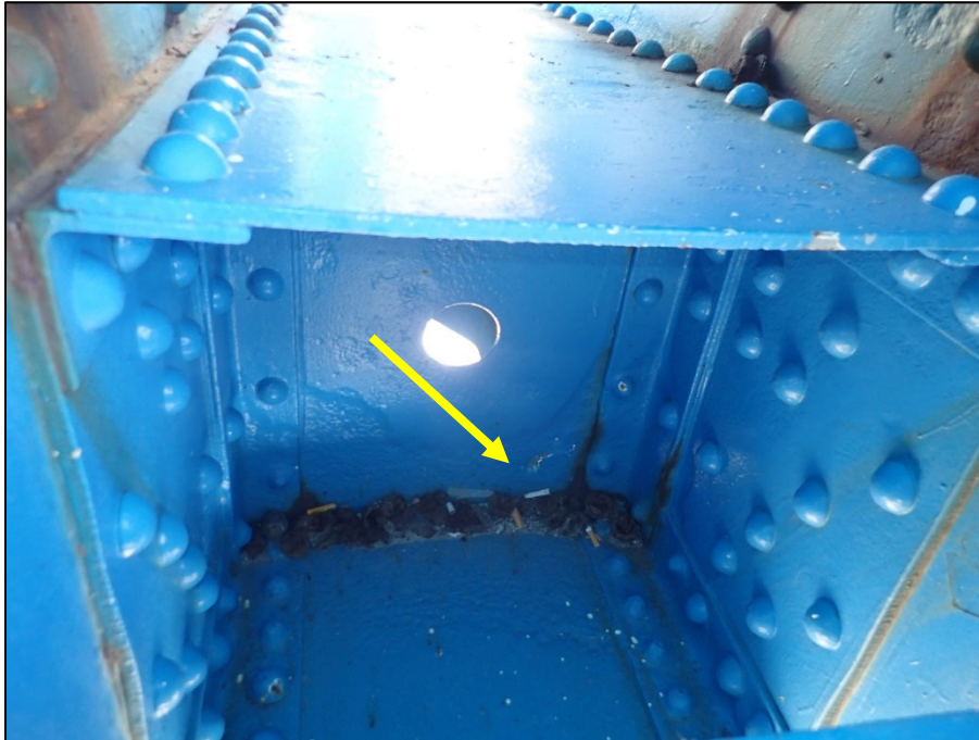
Photo 39 - Unit II, Span 6, North truss at L17; 5" W x 2" H corrosion hole in end plate
