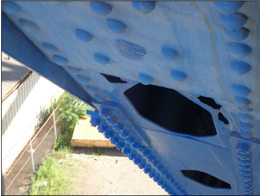
Photo 37 – Unit II, Span 6, North truss under L1; 5" Diameter corrosion hole with 1/4" D pitting
