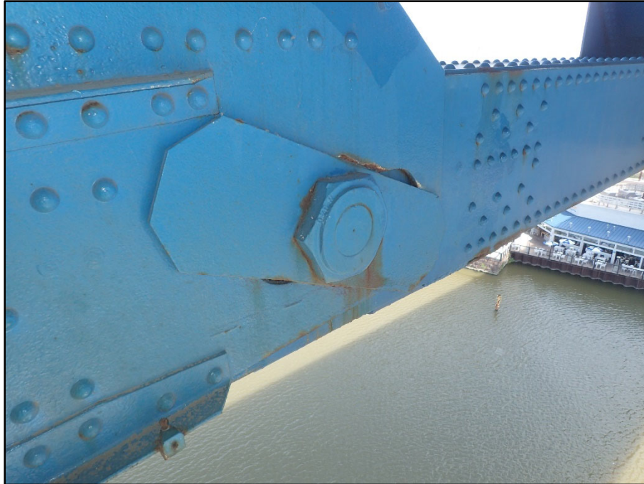
Photo 43 – Unit II, Span 9, North truss at L0; inboard oval pin plate has rotated clockwise
