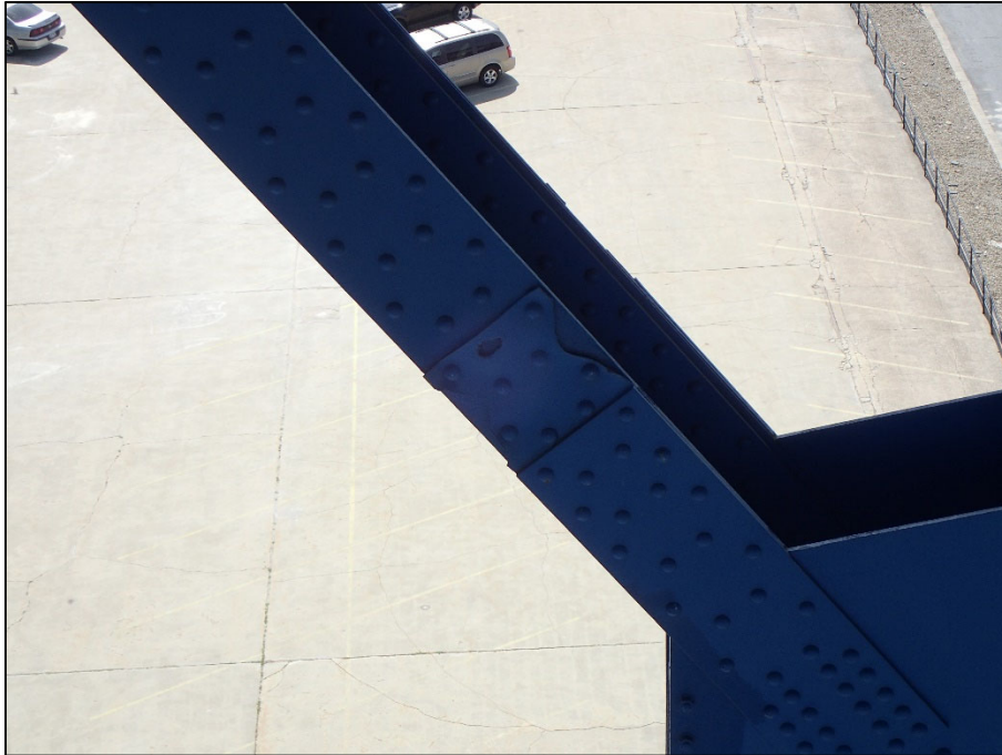
Photo 21 – Unit II, Span 8, South truss near L14; inboard fill plates with painted over corrosion holes
