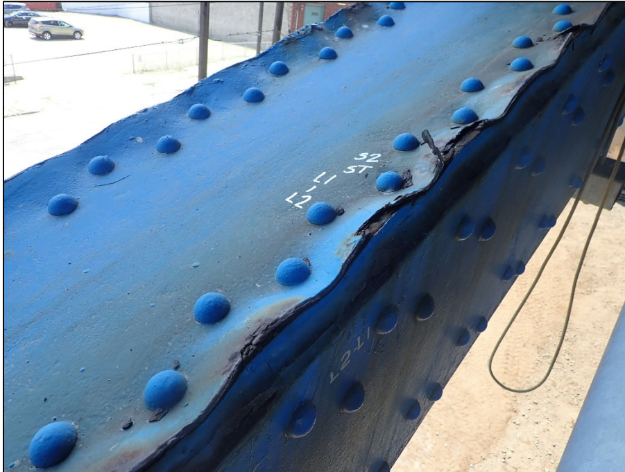
Photo 23 – Unit II, Span 2, South truss, L1L2; up to 2” distortion along inboard and outboard edges of top plate due to reactivated pack rust
