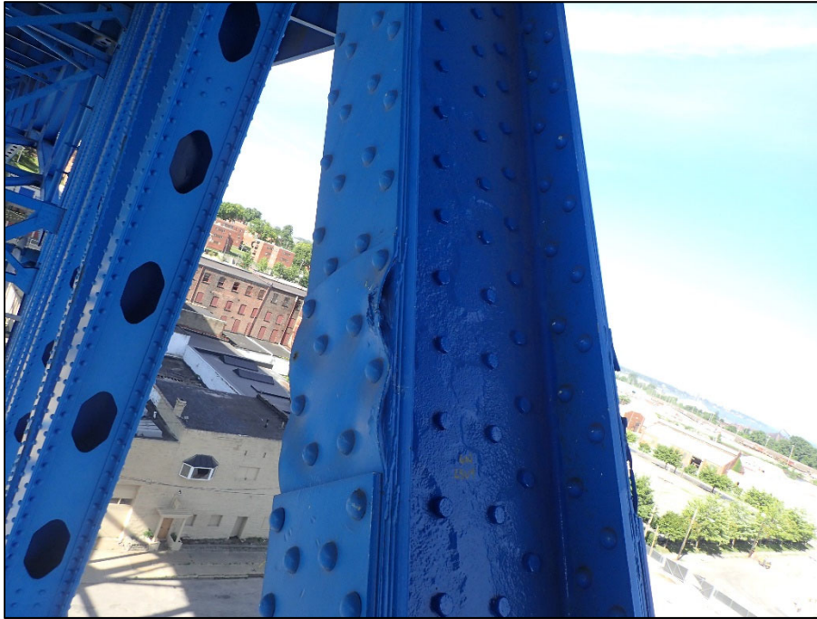
Photo 19 – Unit II, Span 6, North truss at L0U1; 7/16" D painted over pitting along web
