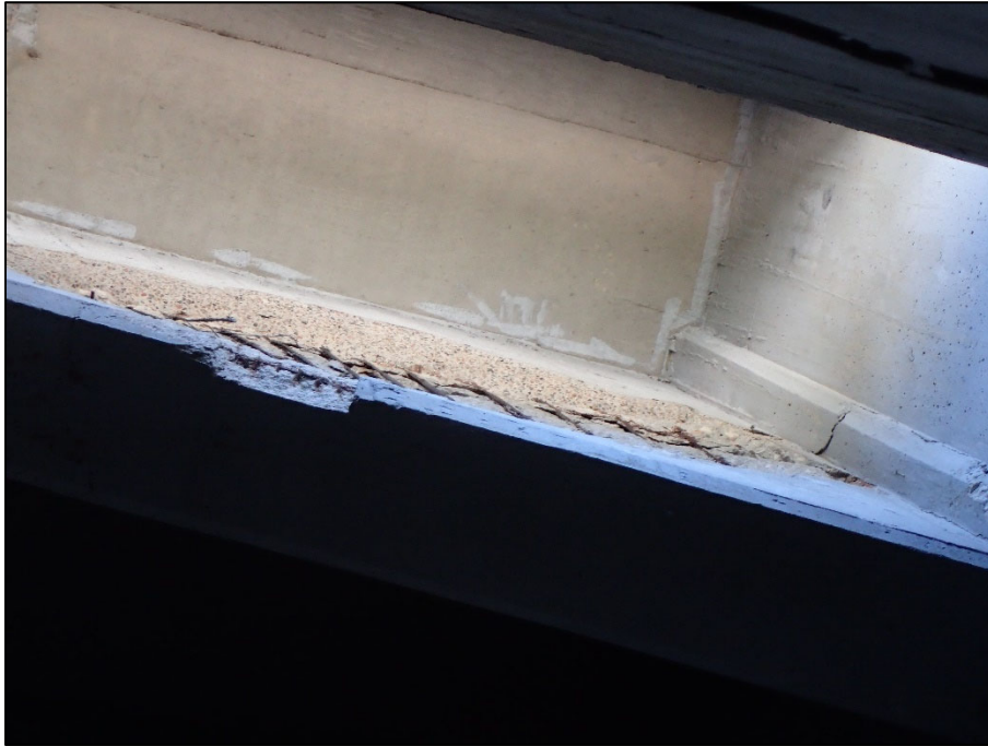
Photo 9 – Unit I, Section P, Frame 1, Floorbeam 2; Full Height x Full Width x 2" D spall with exposed rebar along south end
