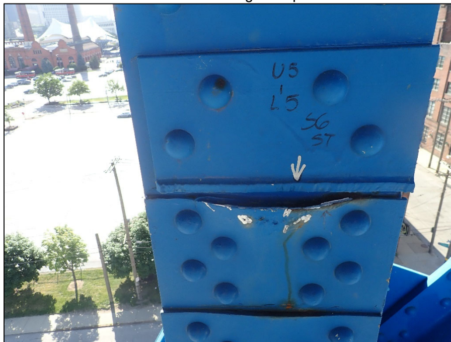
Photo 46 – Unit II, Span 6, South truss at L5; 3" L x 1" H area of section loss with 1 1/8" bow in fill plate
