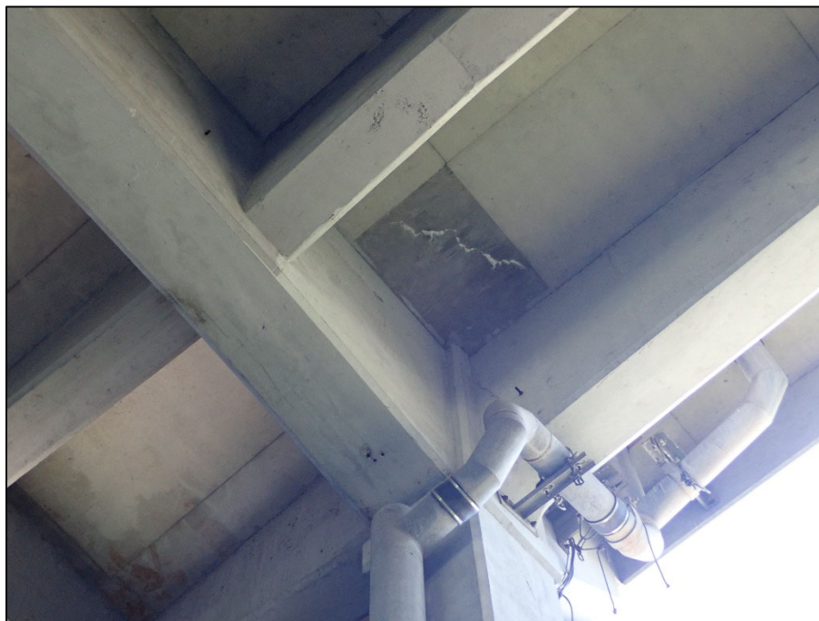
Photo 2 – Unit I, Section P; Transverse cracking with efflorescence
