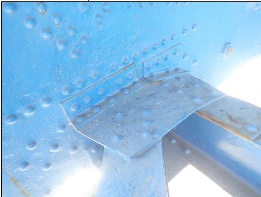
Photo 22 – Unit II, Span 1 South truss at L7; Up to 100% section loss to lower lateral bracing gusset plates
