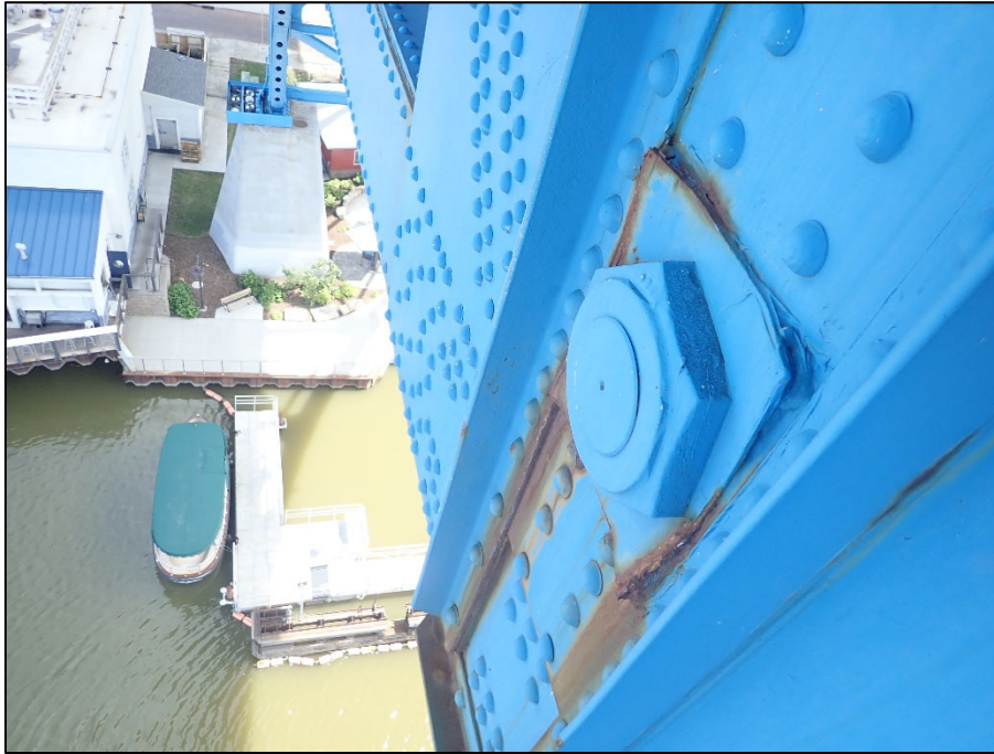
Photo 17 – Unit II, Span 9, North truss at L8; 1" T pack rust between outboard pin plate and vertical
