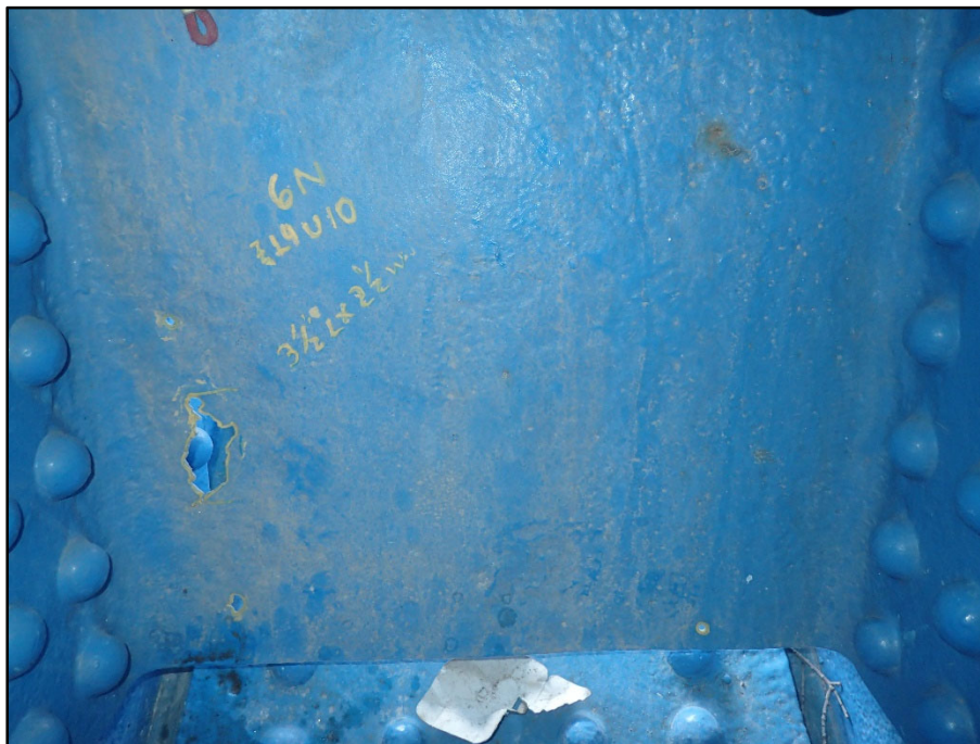
Photo 20 – Unit II, Span 6, North truss at L9; 3-1/2" L x 2-1/2" W corrosion hole with adjacent 1/2" Diameter holes
