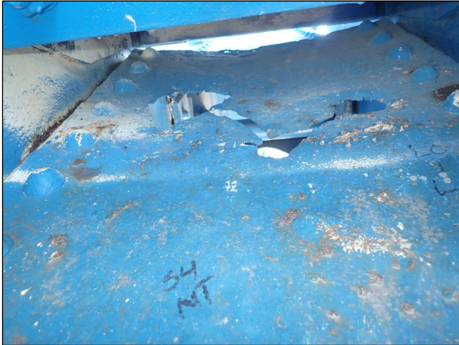
Photo 29 – Unit II, Span 4, North truss at L0; end 16" L with sever painted over dee pitting and 12" W x 16" L corrosion hole
