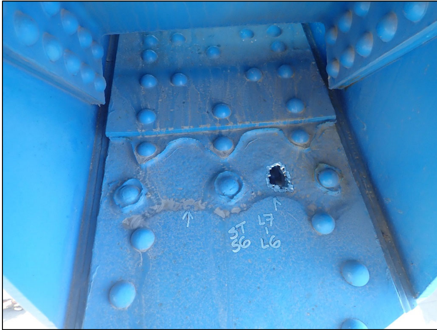
Photo 35 – Unit II, Span 6, South truss at L7; 1/8" T remaining section within 8" L x Full Width with 2" Diameter corrosion hole
