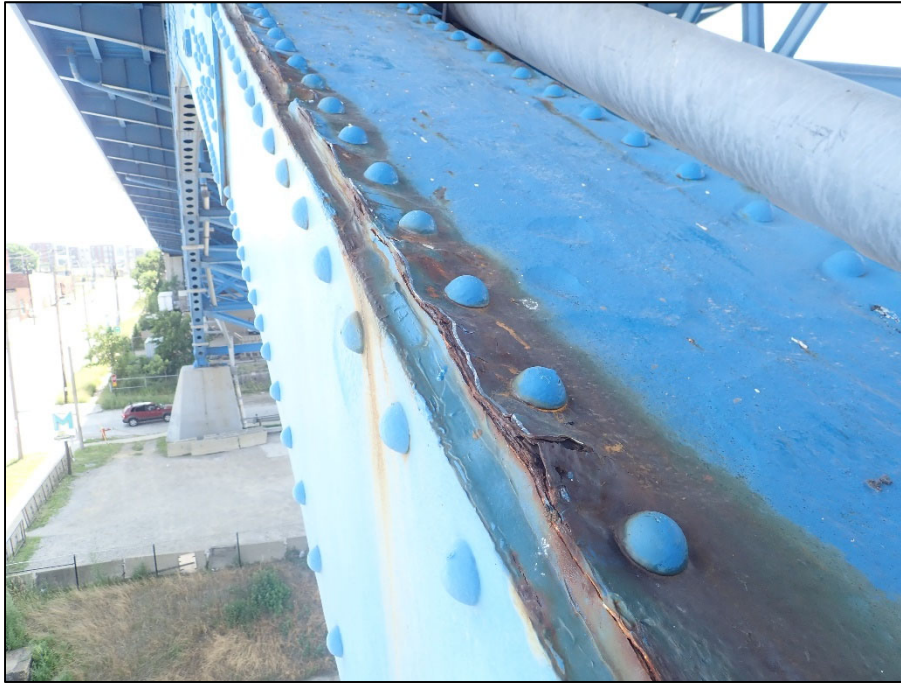
Photo 31 – Unit II, Span 4, South truss at L0L1; 1" T caulked over pack rust along outboard edge of top plate
