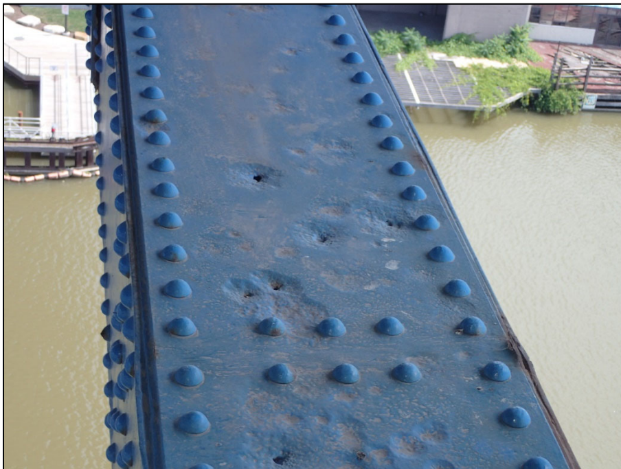
Photo 42 – Unit II, Span 9, South truss along L0L1; Painted over heavy section loss, up to 1/4" D pitting with 1/2" Diameter corrosion holes
