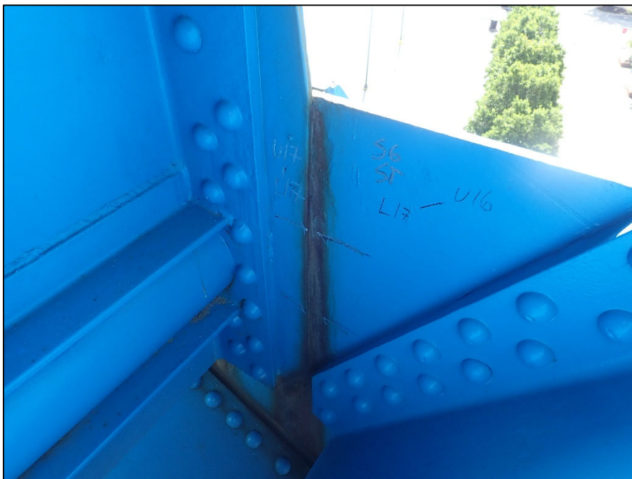
Photo 16 – Unit II, Span 6, South truss at L17; 3/8" T pack rust between outboard gusset and vertical
