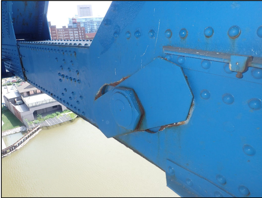
Photo 41 – Unit II, Span 9, South truss at L0; inboard oval pin plate has rotated counterclockwise
