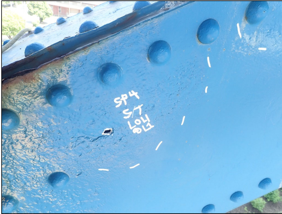
Photo 33 – Unit II, Span 4, South truss near L1; 1" L x 1/2" H painted over corrosion hole in inboard web
