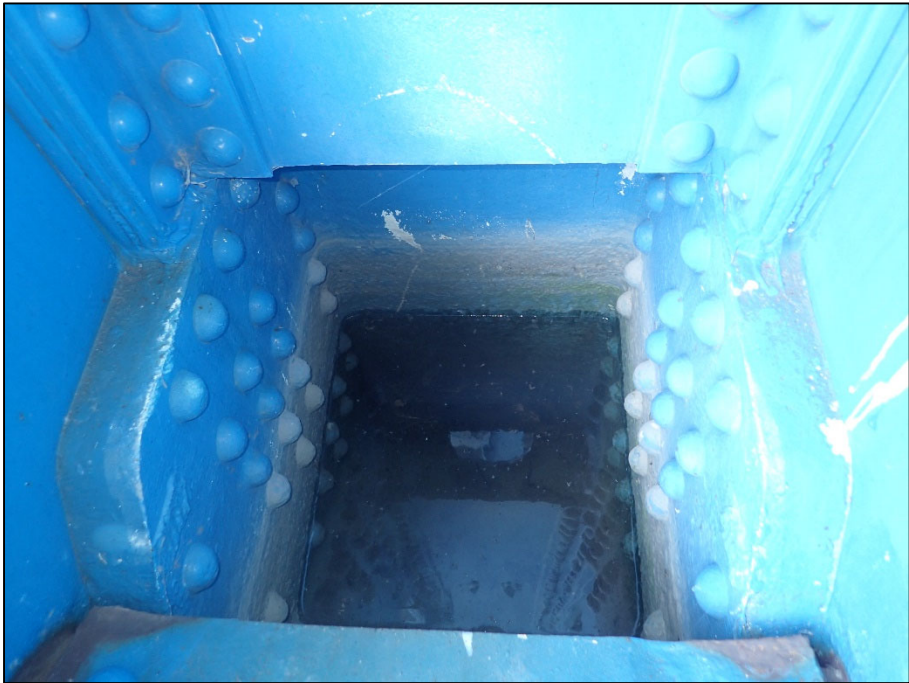
Photo 6 – Unit II, Span 4, L2 bearing; full of water
