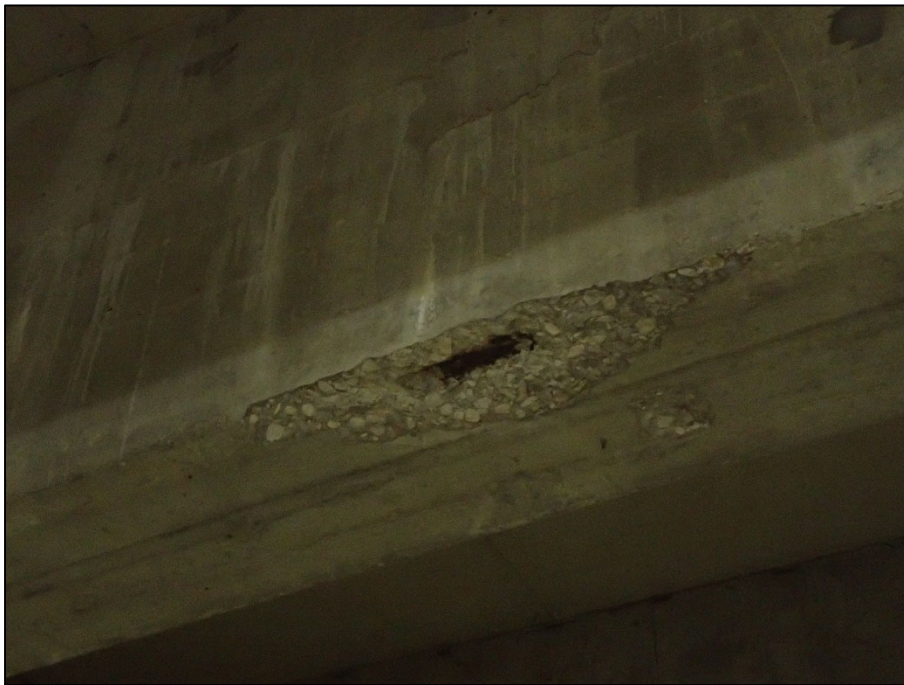
Photo 12 – Unit I, Section M, Frame 12; 2' L x 6" W x 3" D spall
