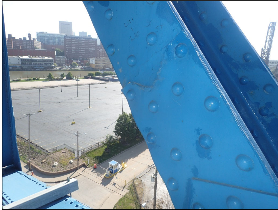
Photo 47 – Unit II, Span 6, South truss at L10; interior fill plate with painted over section loss and corrosion holes in fill plates
