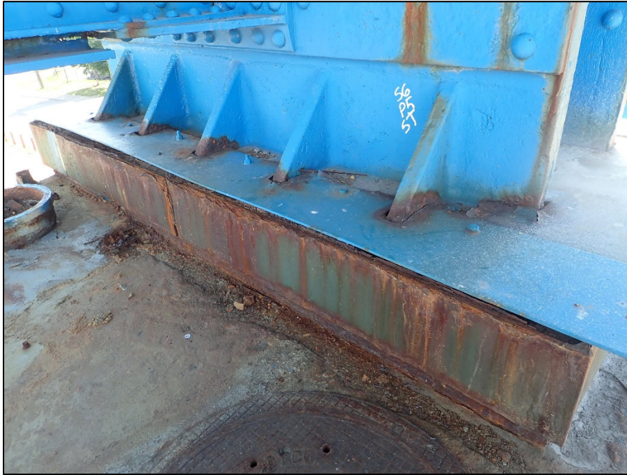
Photo 7 – Unit II, Pier 5, South bearing; moderate surface corrosion along vertical steel box sides
