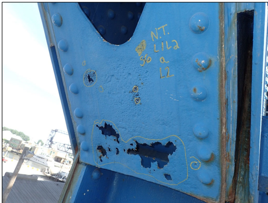
Photo 38 - Unit II, Span 6, North truss at L1; 10" L x 4" W corrosion hole
