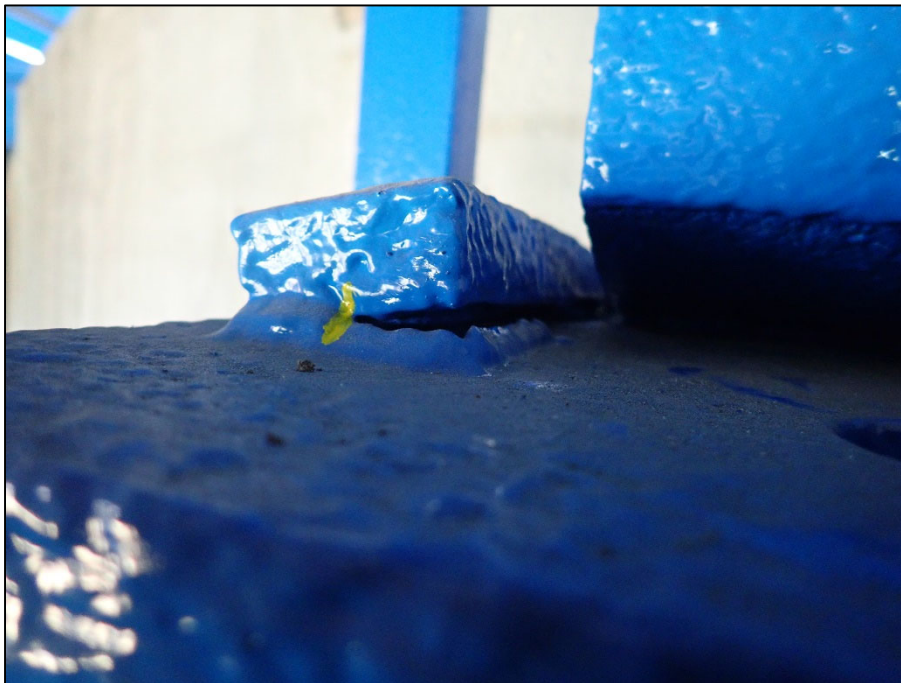
Photo 8 – Unit I, Section N, Floorbeam 8; south guide bar of north bearing is cracked
