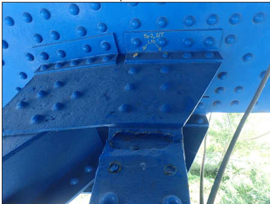
Photo 24 – Unit II, Span 2, South truss, L10; Multiple corrosion holes in lower lateral bracing
