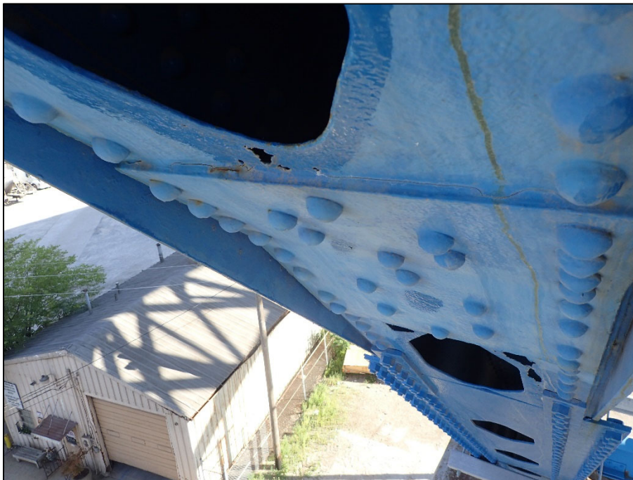
Photo 36 - Unit II, Span 6, North truss at L2; 8" L x 1-1/2" W corrosion hole in bottom flange
