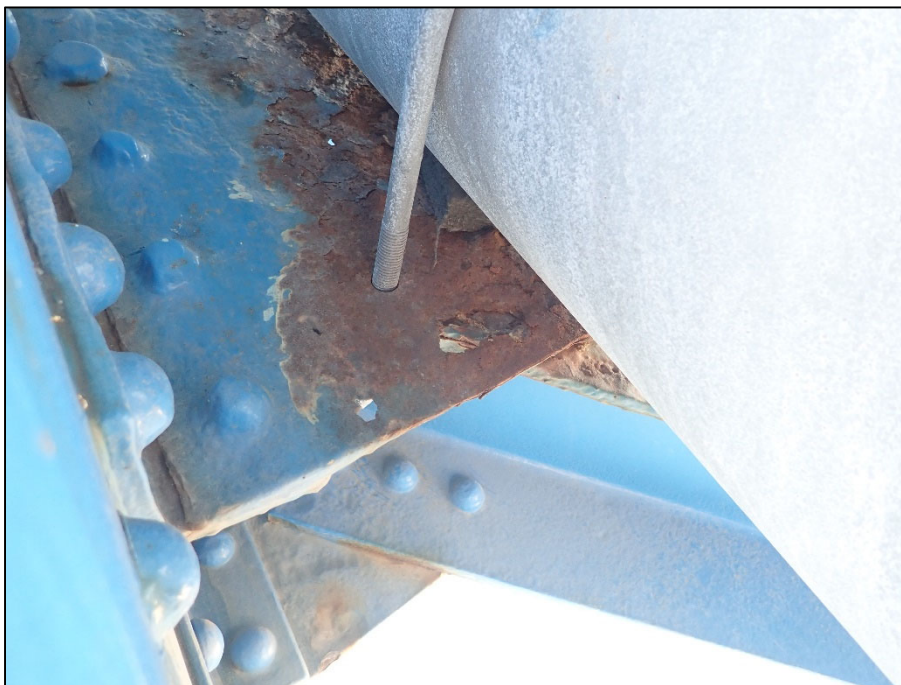
Photo 32 – Unit II, Span 4, South truss; Corrosion holes in lower lateral bracing gusset plate
