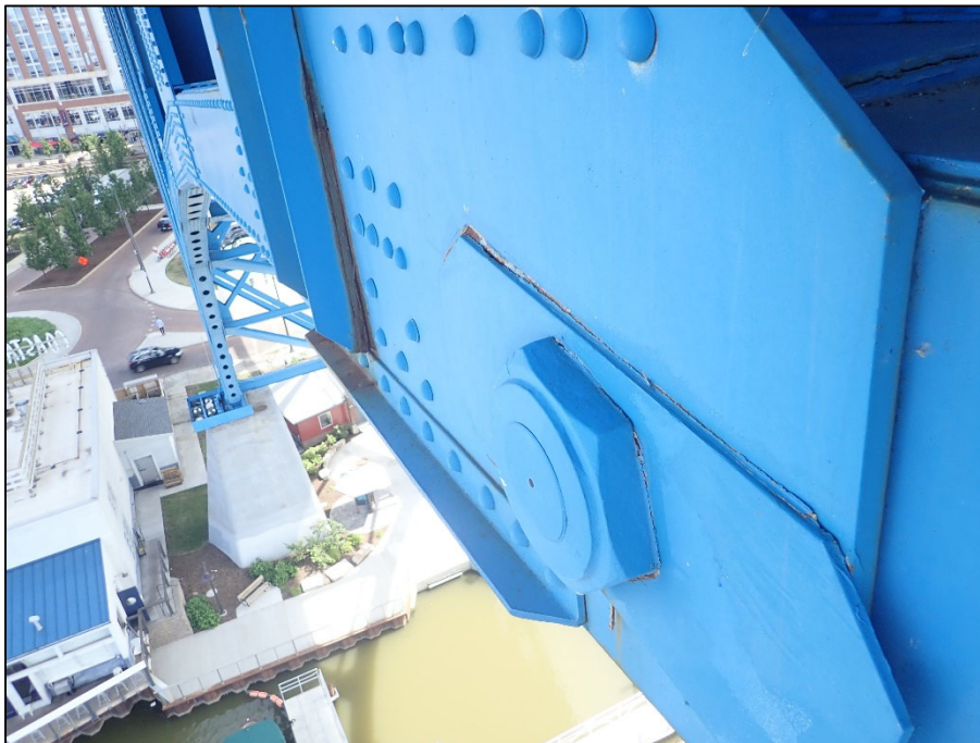
Photo 18 – Unit II, Span 6, South truss at L5; deteriorated caulk along outboard face
