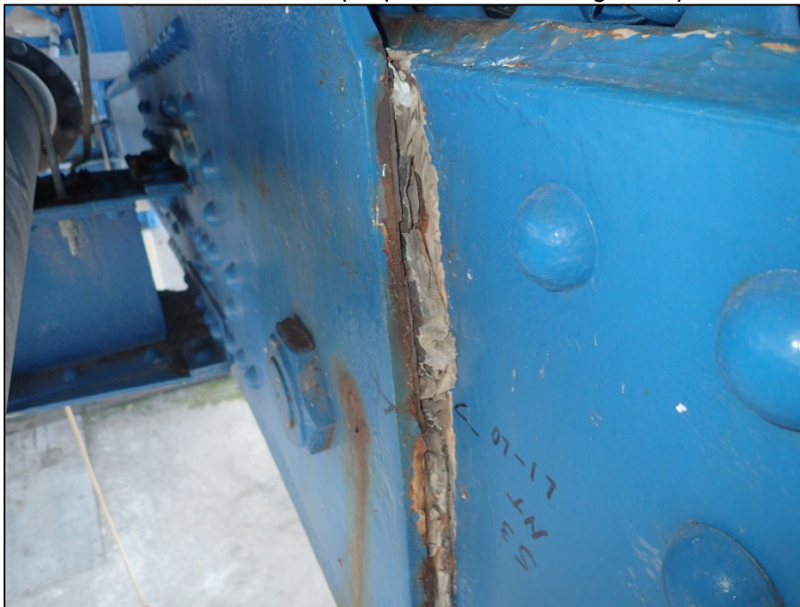
Photo 28 – Unit II, Span 3, North truss at L0; 1" T pack rust between lower chord and interior gusset plate
