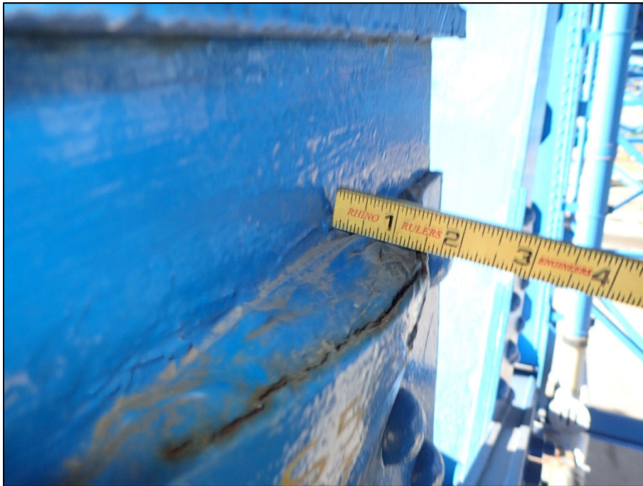
Photo 15 – Unit II, Span 5, South truss at L1; 1-5/8" T painted over pack rust on inboard fill plate
