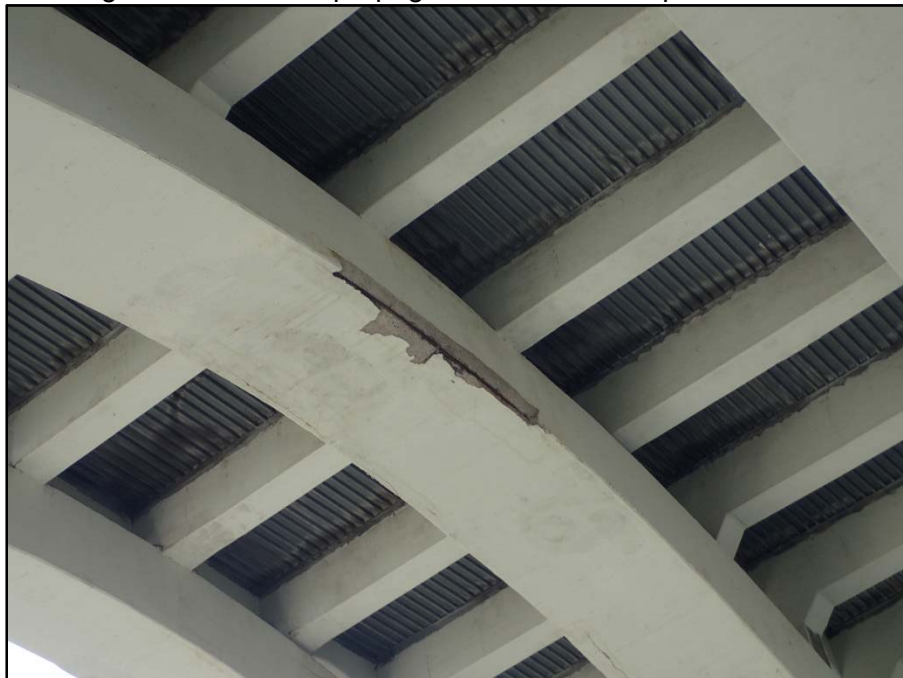
Photo 19 – Span 7 South Interior Arch Rib; lower north corner near apex has an unrepaired spall with exposed reinforcing
