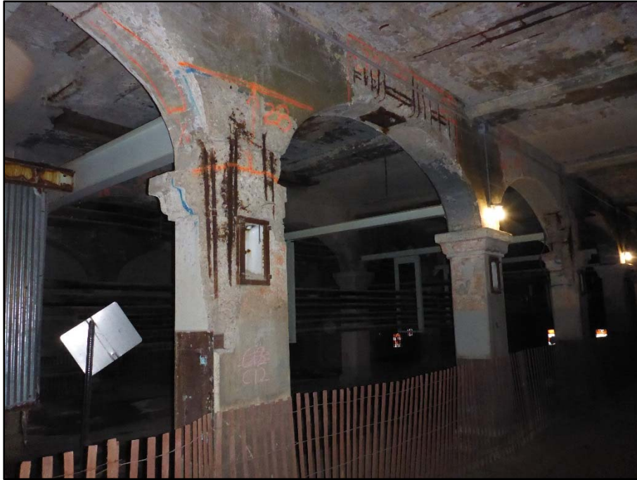
Photo 40 – West Station Columns and Arches; heavily deteriorated with exposed reinforcing and efflorescence
