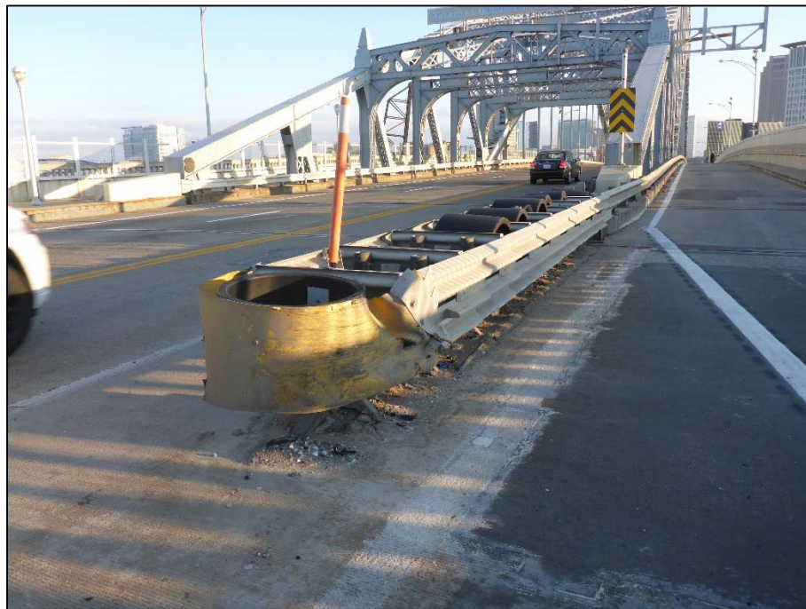
Photo 12 – Span 3 south attenuator; minor impact damage
