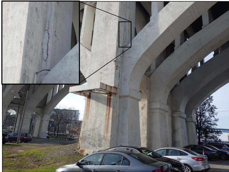
Photo 43 – Pier 8 South Exterior Column, East Face; 6' H x 3'W delamination above parked cars
