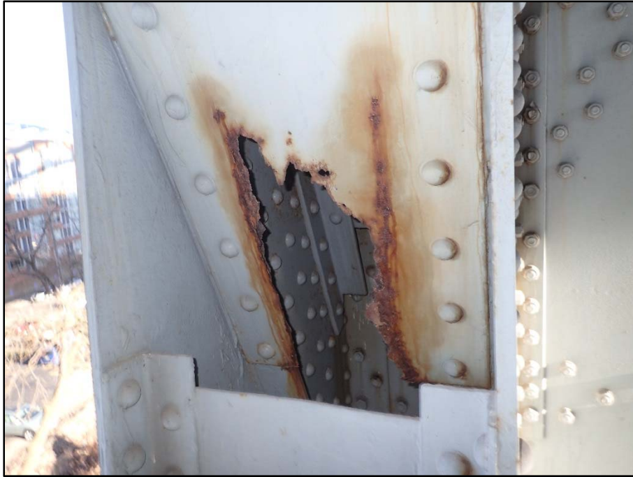
Photo 34 – Span 4 North Truss L2 lower batten plate; 20" L x 8" W corrosion hole
