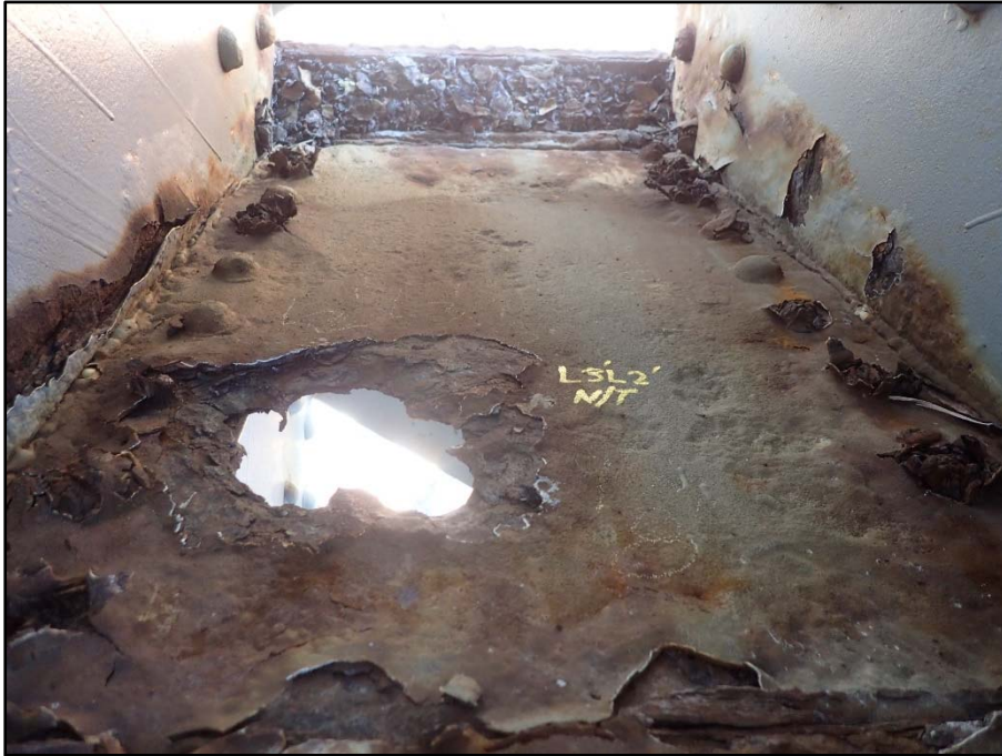
Photo 30 – Span 4 North Truss L3'L2' diaphragm; corrosion hole
