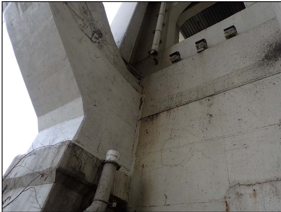
Photo 10 – Pier 1 south downspout; missing 15' section of PVC pipe
