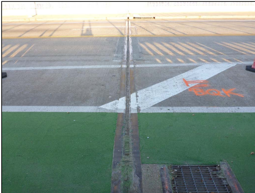
Photo 6 – Typical expansion joint condition
