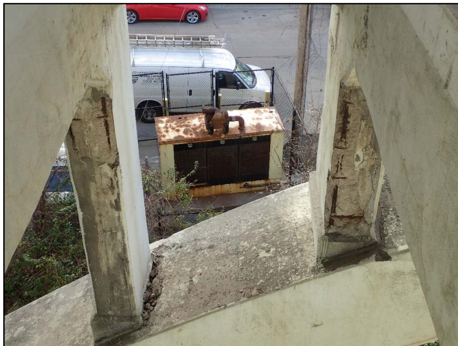
Photo 21 – Span 2 North Exterior lower columns 3 and 4; south faces have up to full height spalling with corroded reinforcing
