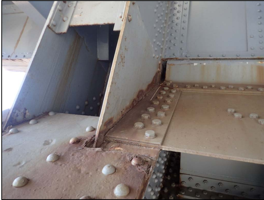
Photo 32 – Span 4 North Truss L3 south gusset above L2L3; Active laminar corrosion and pitting up to 3/16" D
