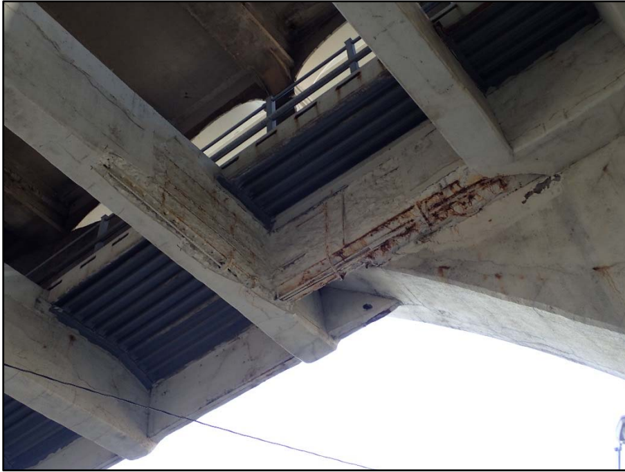
Photo 24 – Span 12, lower deck floorbeams; multiple floorbeams have chipped off concrete with exposed, painted reinforcing
