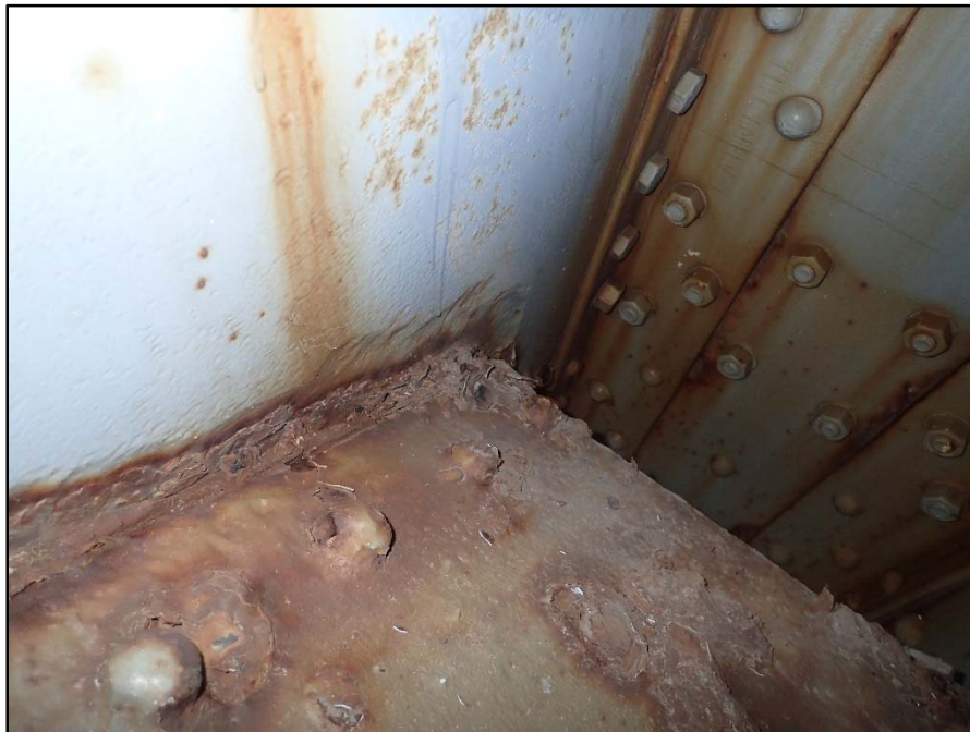
Photo 33 – Span 4 North Truss L2 South Gusset, North Face; 2' L x up to 3' H x up to 1/4" D pitting with reactivating laminar corrosion
