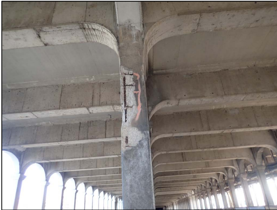
Photo 22 – Span 8 North Interior Upper Column 2; 4' H x 4" D corner spall on the northeast corner of the column with exposed reinforcing
