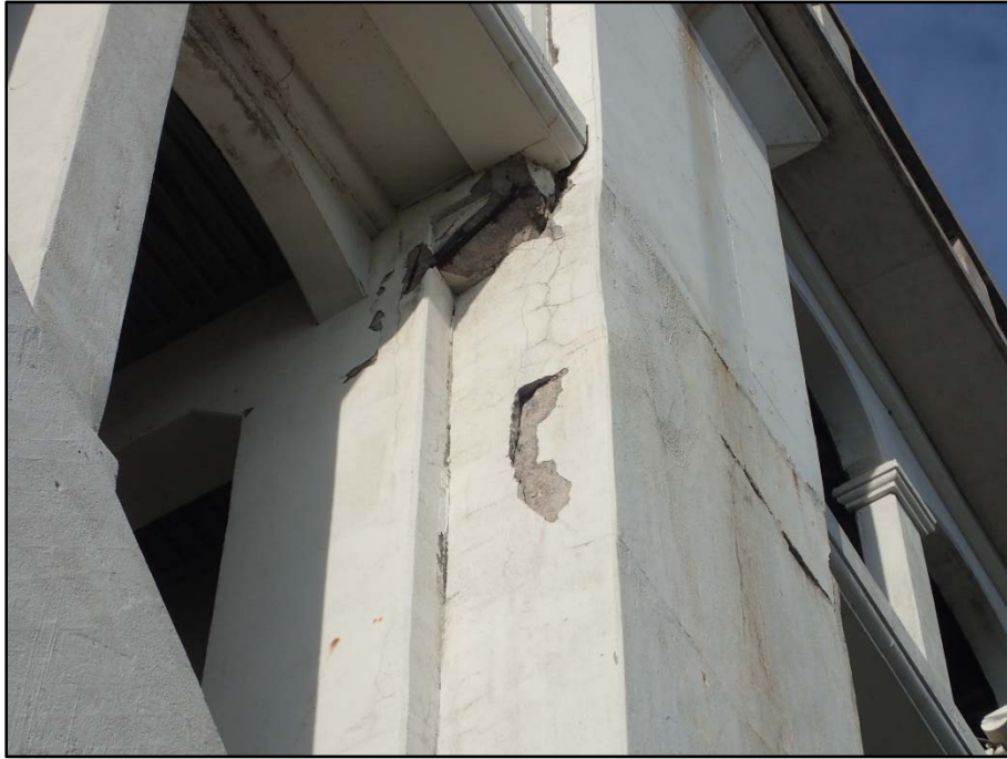
Photo 44 – Pier 8 South Exterior Column, West Face; 4' H x 4' W x 10" D spall
