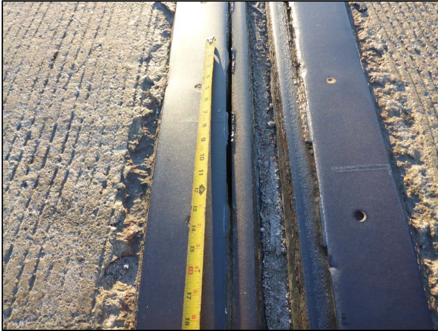
Photo 17 – Tower B expansion joint, left westbound lane; Pack rust has broken fillet welds. Snow plow damage is present.
