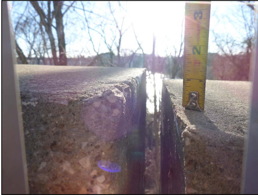
Photo 7 – South top railing at Tower A; vertically misaligned 7/8” at railing joint
