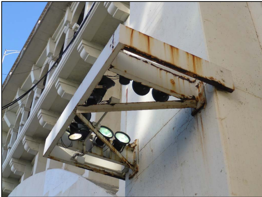
Photo 39 – Pier 2 North Face; architectural lighting brackets are corroding
