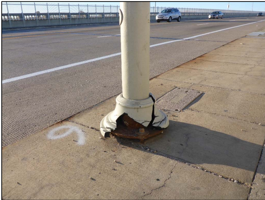
Photo 16 – Span 11, North sidewalk; broken light pole base
