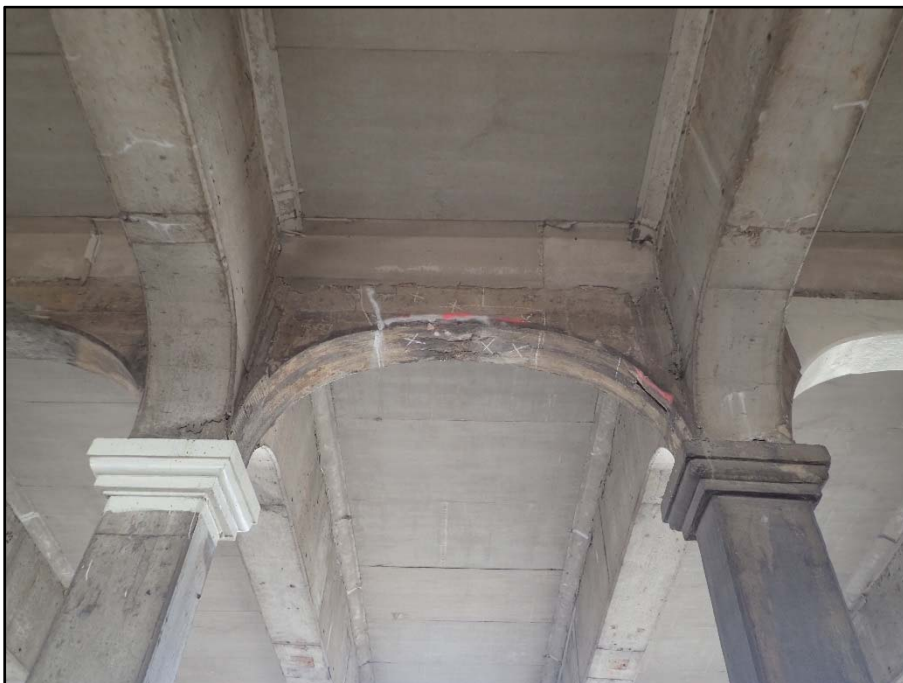
Photo 25 – Span 3 North Interior Arch between upper deck Columns 10 & 11; arch is cracked and delaminated with efflorescence
