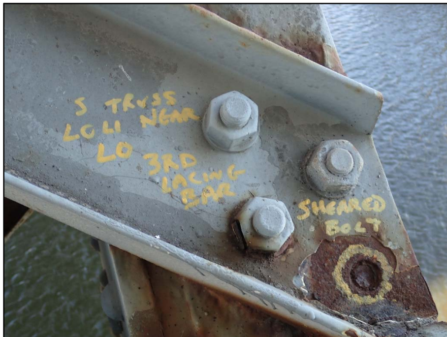
Photo 31 – Span 4 South Truss L0L1 near L0; fractured bolt on top lacing channel connection along top flange
