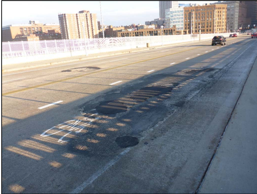
Photo 15 – Span 8 eastbound lane; 36' L deteriorating asphalt patch
