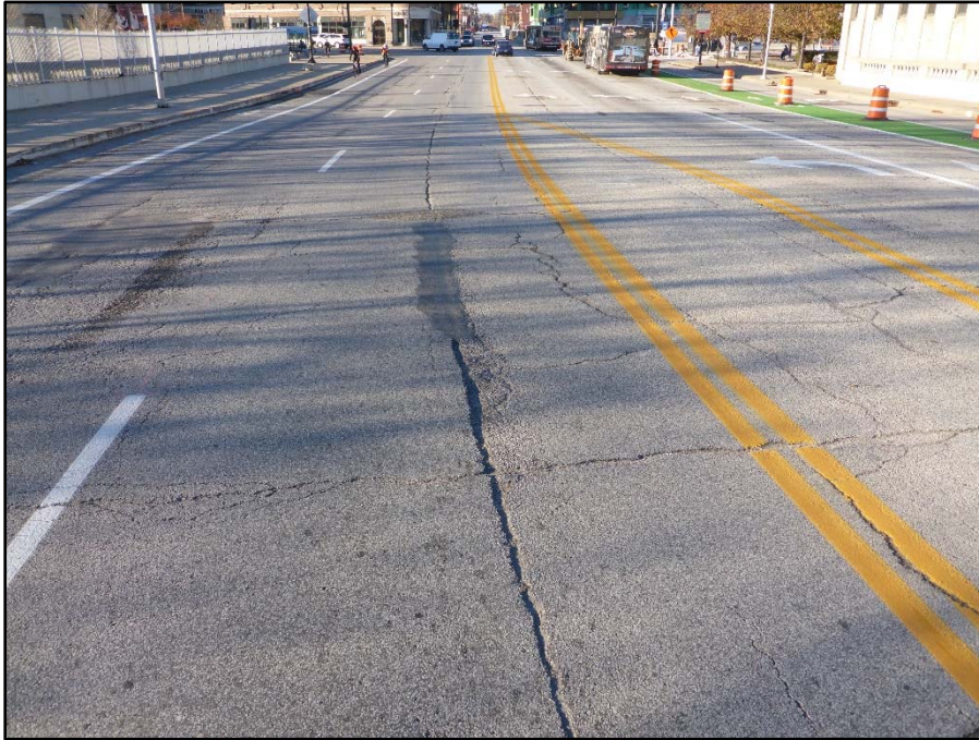
Photo 9 – West Station wearing surface; heavy map cracking and patching throughout
