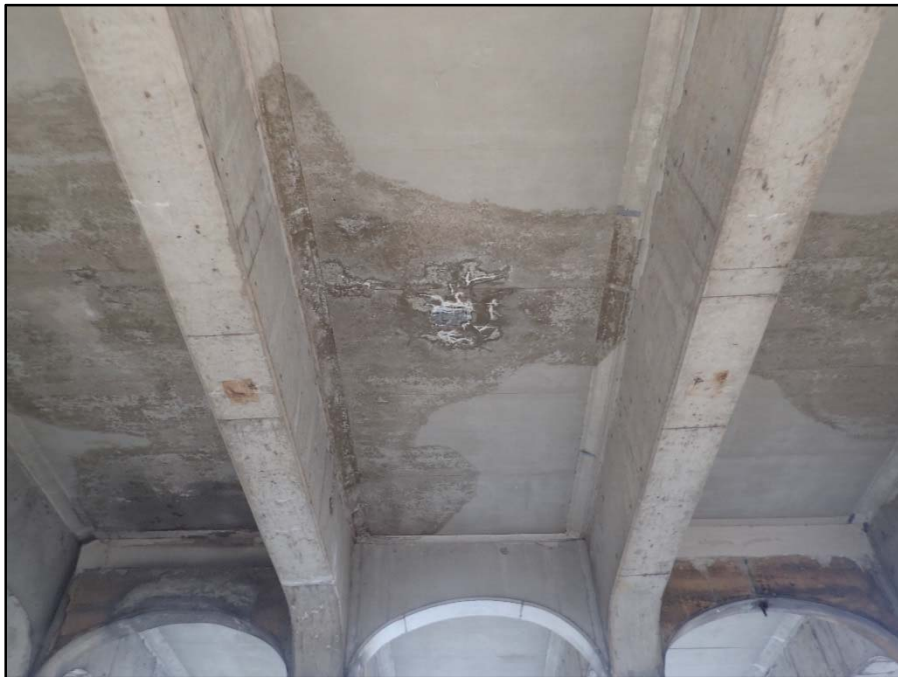
Photo 14 – Upper Deck, Span 7, Panel 4 center bay; local area of efflorescence
