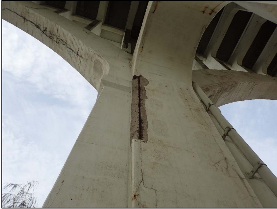
Photo 42 – Pier 5 North Exterior Column; 10' H x 6" D corner spall with exposed reinforcing
