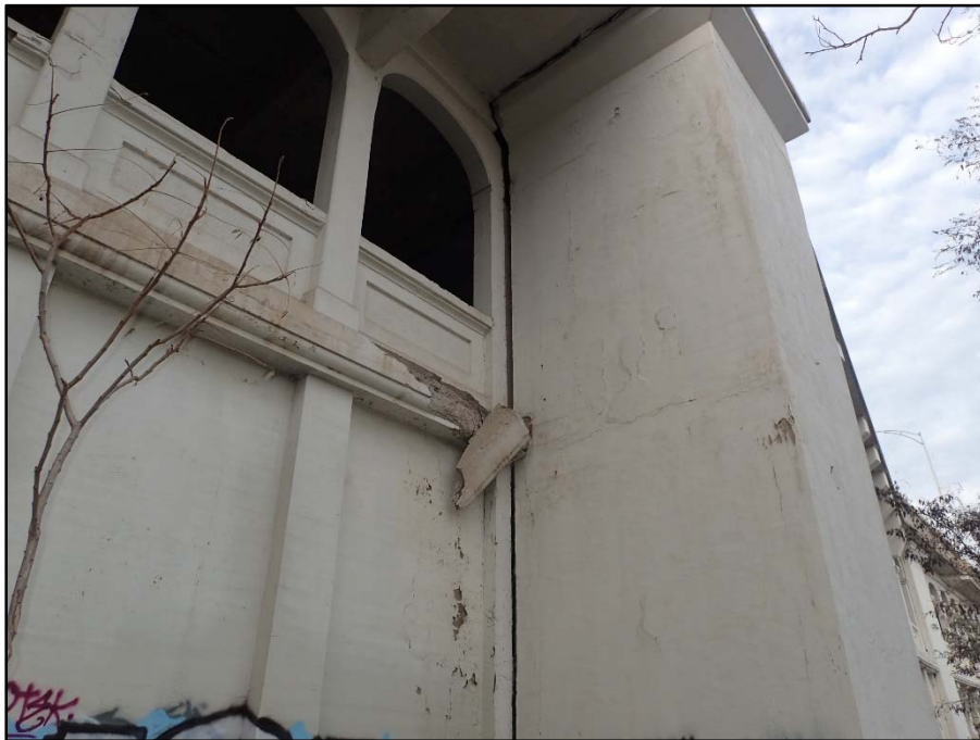
Photo 45 – Tower B South side; rotated outwards and fractured at the interface with the upper deck
