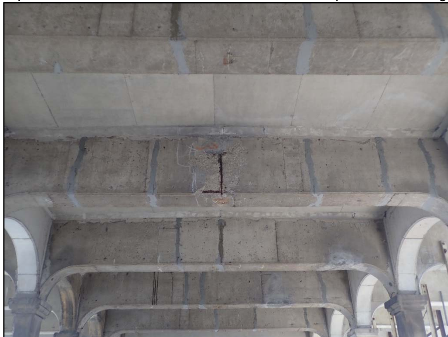
Photo 23 – Span 5 Upper Deck Floorbeam 11 west face between interior arches; Full height x 3' W x 4" D spall with exposed rebar
