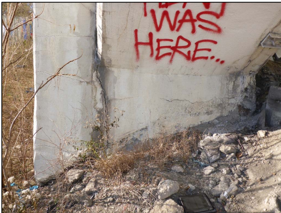
Photo 41 – West Abutment Below South Exterior Arch; 1/4" W vertical crack
