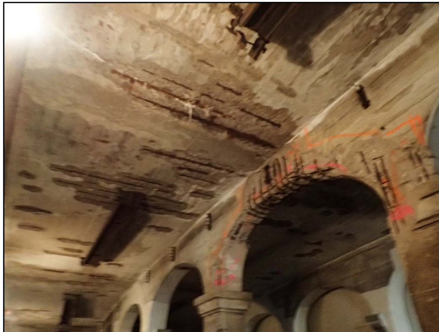
Photo 8 – West tunnels upper deck with heavy efflorescence, cracking, delaminations, and spalls with corroded reinforcing steel
