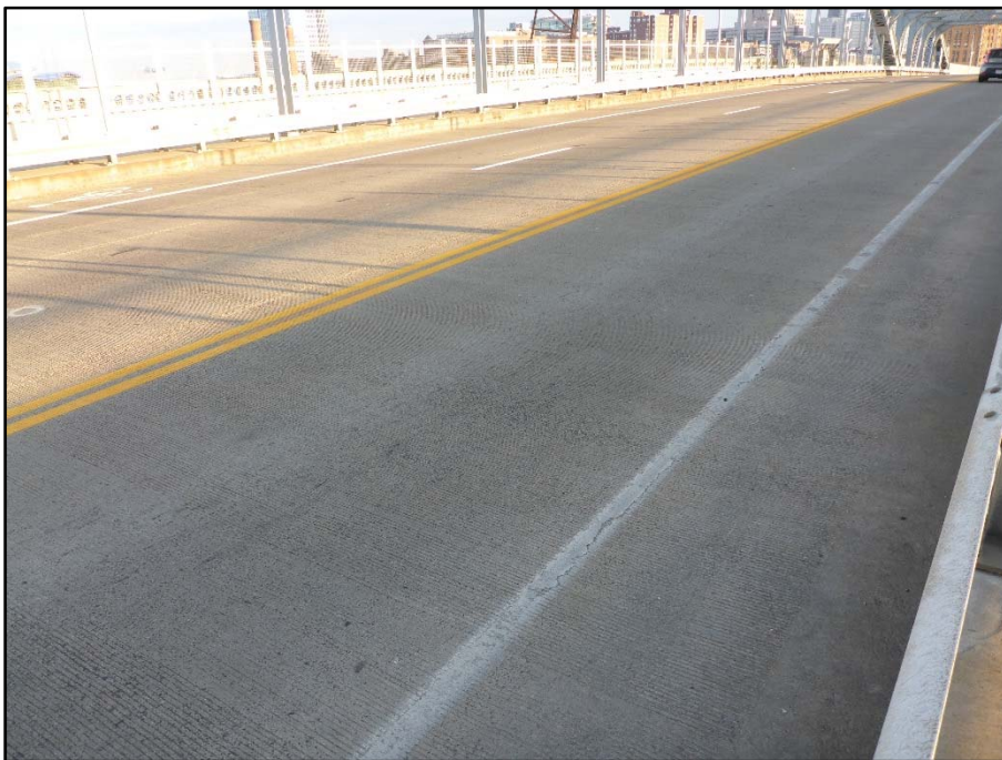
Photo 4 – Typical upper deck wearing surface condition
