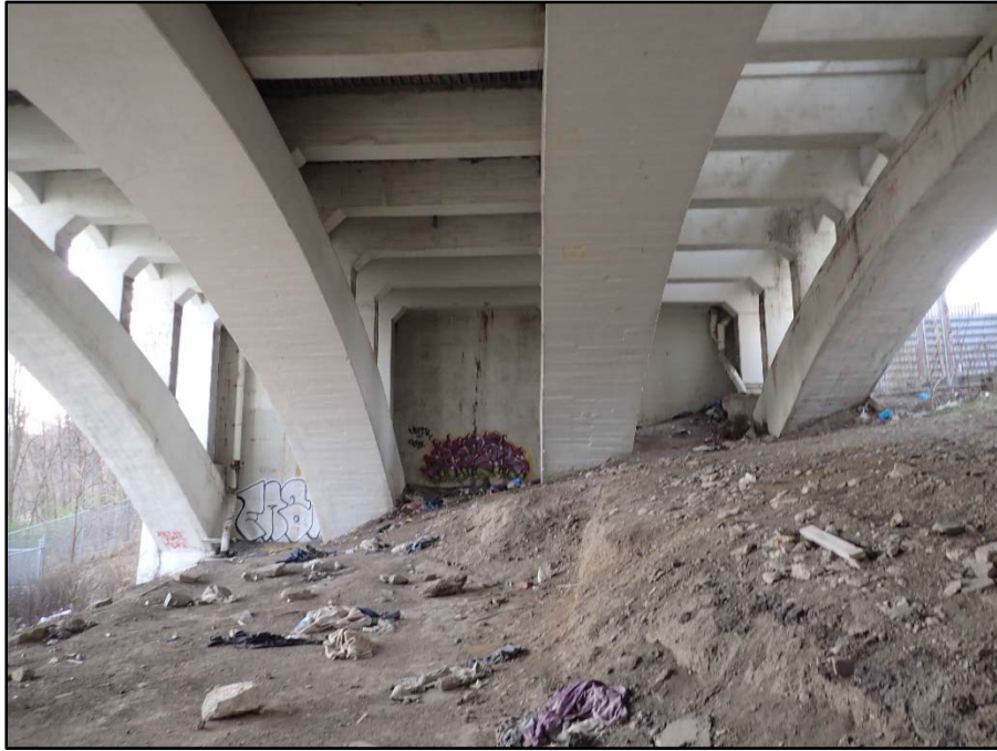
Photo 38 – West Abutment typical condition
