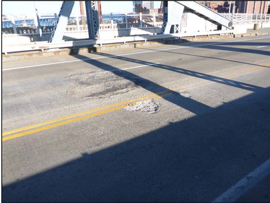
Photo 13 – East end of Span 4; deteriorating 6' Diameter patch with adjacent 2' Diameter x 1-1/2" D pothole
