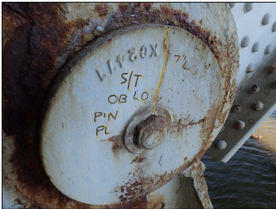
Photo 35 – Span 4 South Truss L0 Outboard Pin Cover Plate; non-structural plate with 7" L crack
