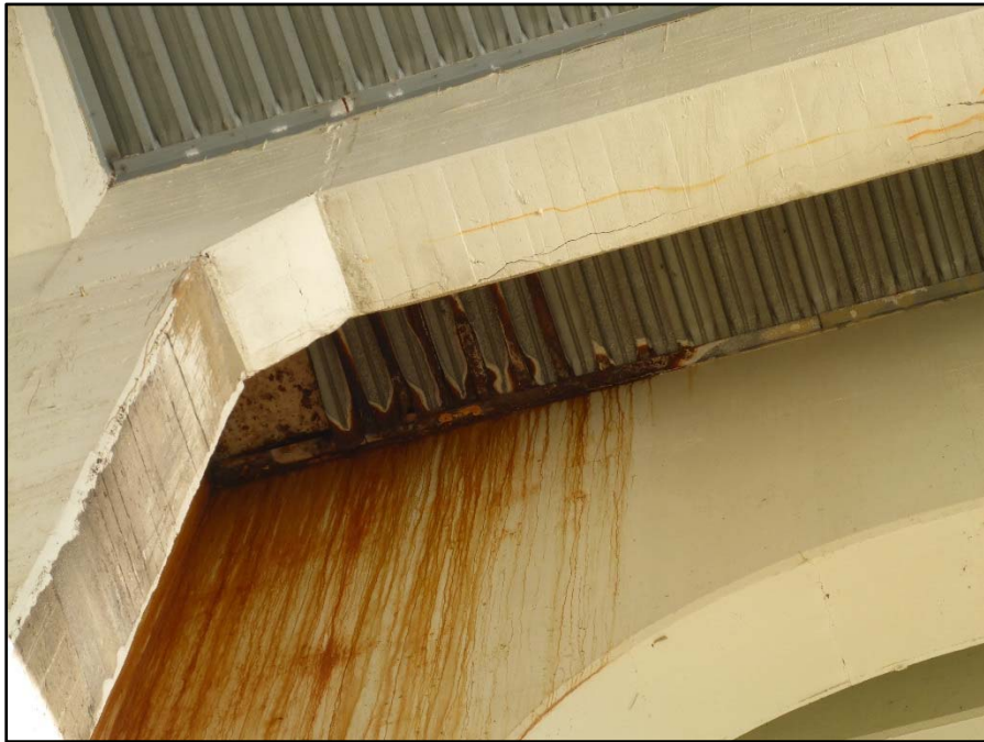
Photo 11 – Span 2, Panel 15 center bay; SIP forms exhibit severe corrosion that is staining the west face of Pier 2
