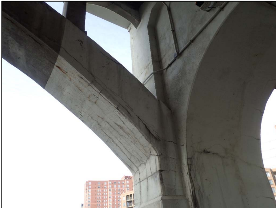
Photo 20 – Span 11 North Exterior Arch, south face; crack extending from Pier 11 up 1/4 length of the arch
