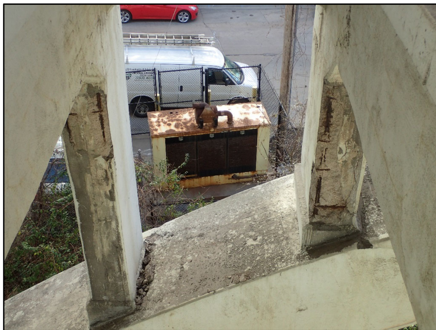
Photo 21 – Span 2 North Exterior lower columns 3 and 4; south faces have up to full height spalling with corroded reinforcing
