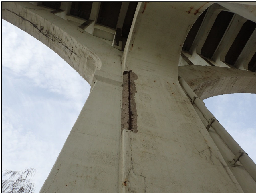
Photo 43 – Pier 5 North Exterior Column; 10' H x 6" D corner spall with exposed reinforcing
