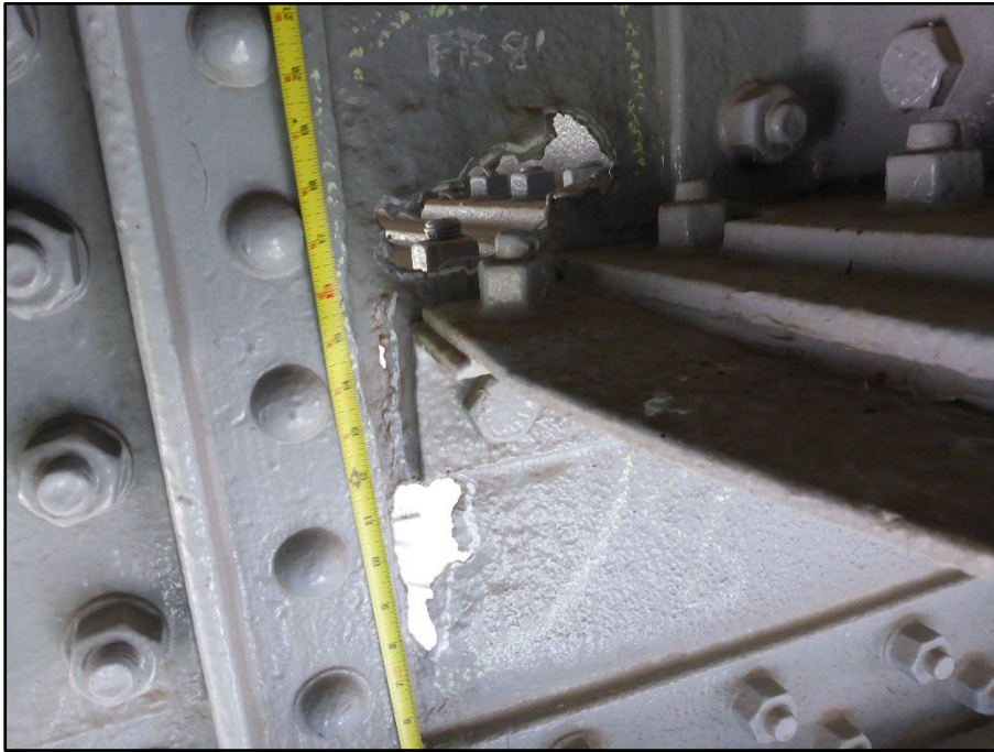
Photo 32 – Span 4 Upper Deck Floorbeam 8'; corrosion hole below the upper deck lateral bracing gusset plate on the north arch
