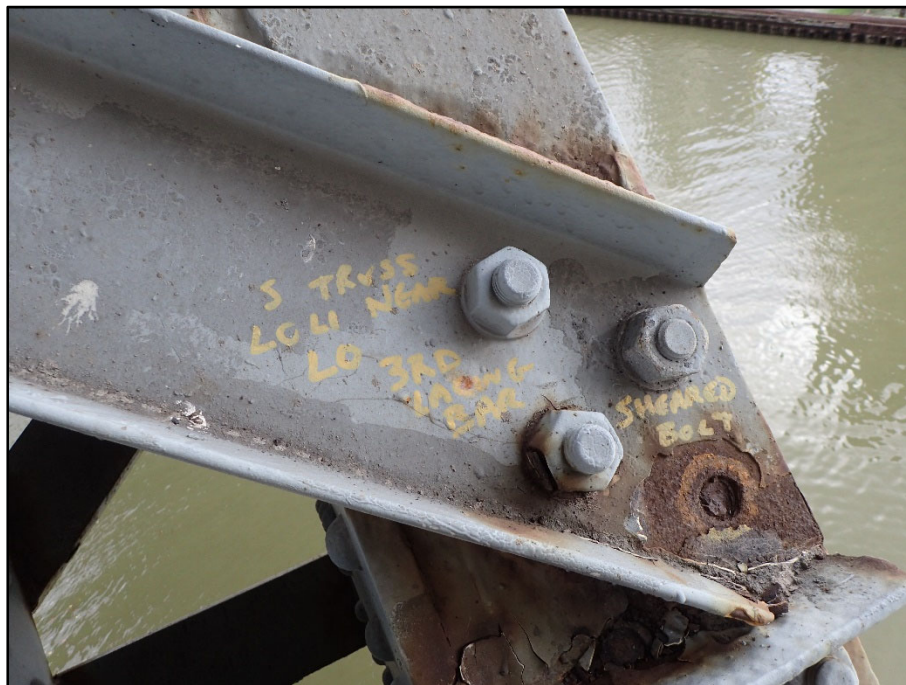
Photo 35 – Span 4 South Truss L0L1 near L0; fractured bolt on top lacing channel connection along top flange
