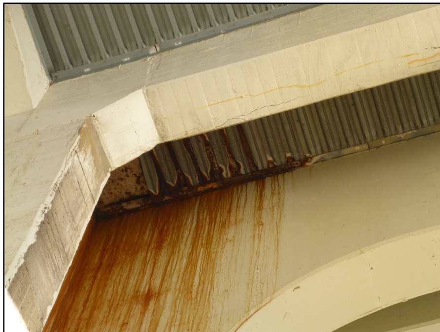
Photo 12 – Span 2, Panel 15 center bay; SIP forms exhibit severe corrosion that is staining the west face of Pier 2
