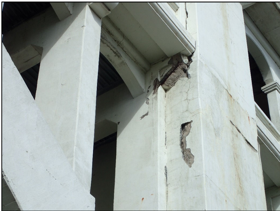
Photo 45 – Pier 8 South Exterior Column, west Face; 4' H x 4' W x 10" D spall
