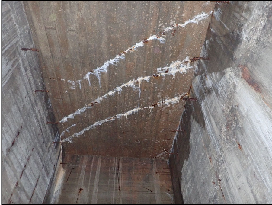
Photo 48 – West Abutment, Chamber 1S, ceiling; typical cracks with efflorescence and moisture
