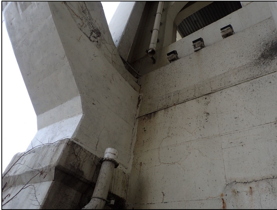
Photo 11 – Pier 1 south downspout; missing 15' section of PVC pipe
