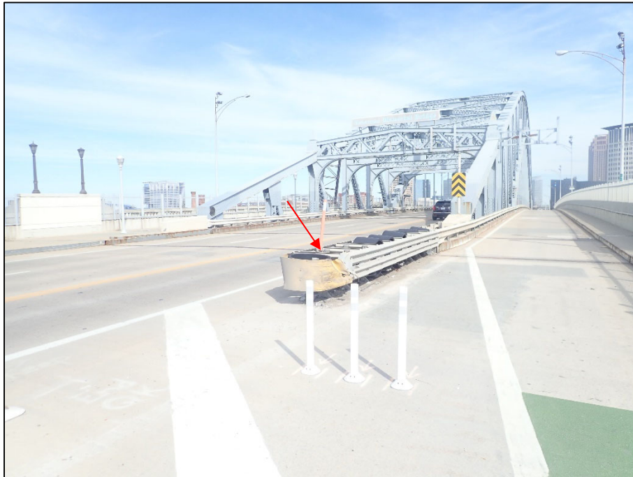
Photo 13 – Span 3 south attenuator; minor impact damage
