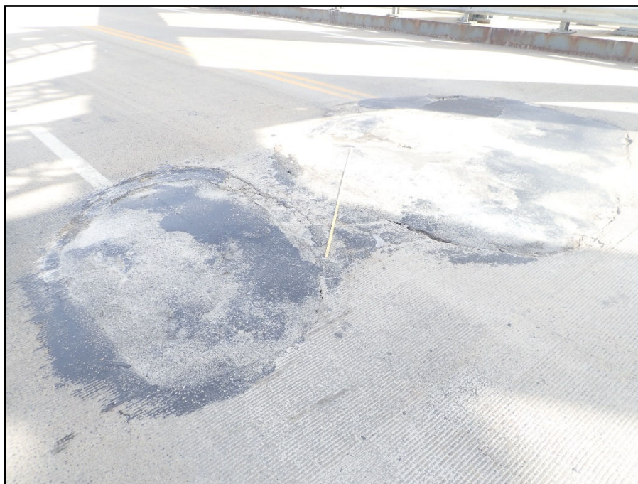
Photo 14 – East end of Span 4; deteriorating 12' L x 18' W x 1" D patch
