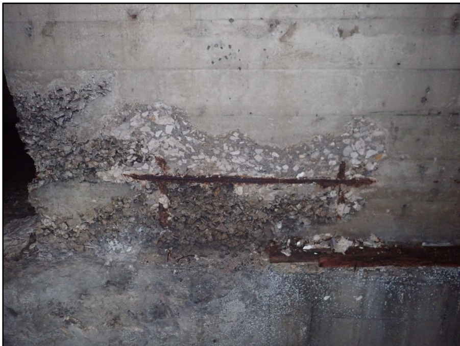
Photo 49 – West Abutment, Chamber 7, west wall; 4' L x 20" H x 1" D spall with exposed reinforcing
