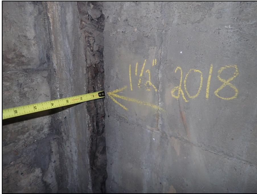
Photo 46 – West Abutment, Chamber 9S, south wall; 1-1/2” rotation towards the south
