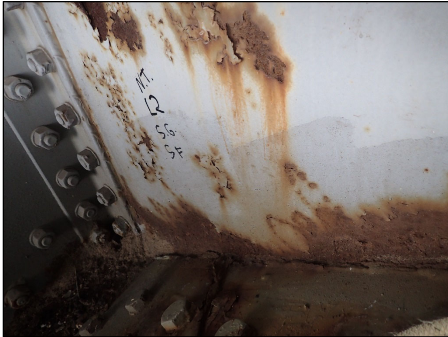
Photo 28 – Span 4 North Truss L2 South Gusset, North Face; 2' L x up to 3" H x up to 1/4" D pitting with reactivating laminar corrosion
