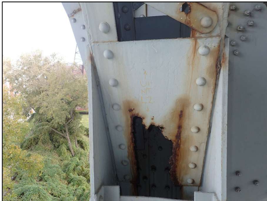
Photo 29 – Span 4 North Truss L2 lower batten plate; 20" L x Full Width corrosion hole
