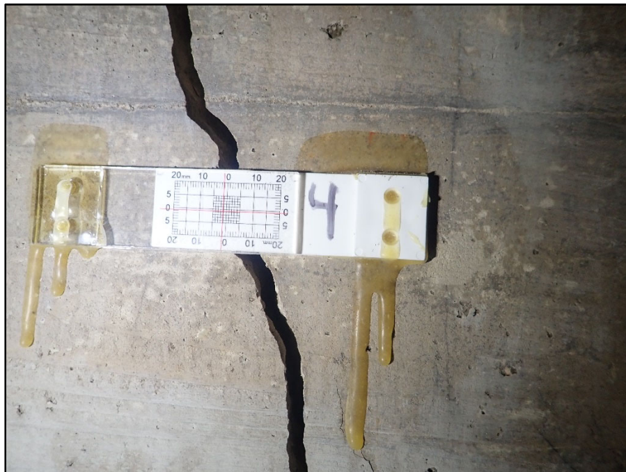
Photo 47 – West Abutment, Chamber 6S, west wall; crack gauge
