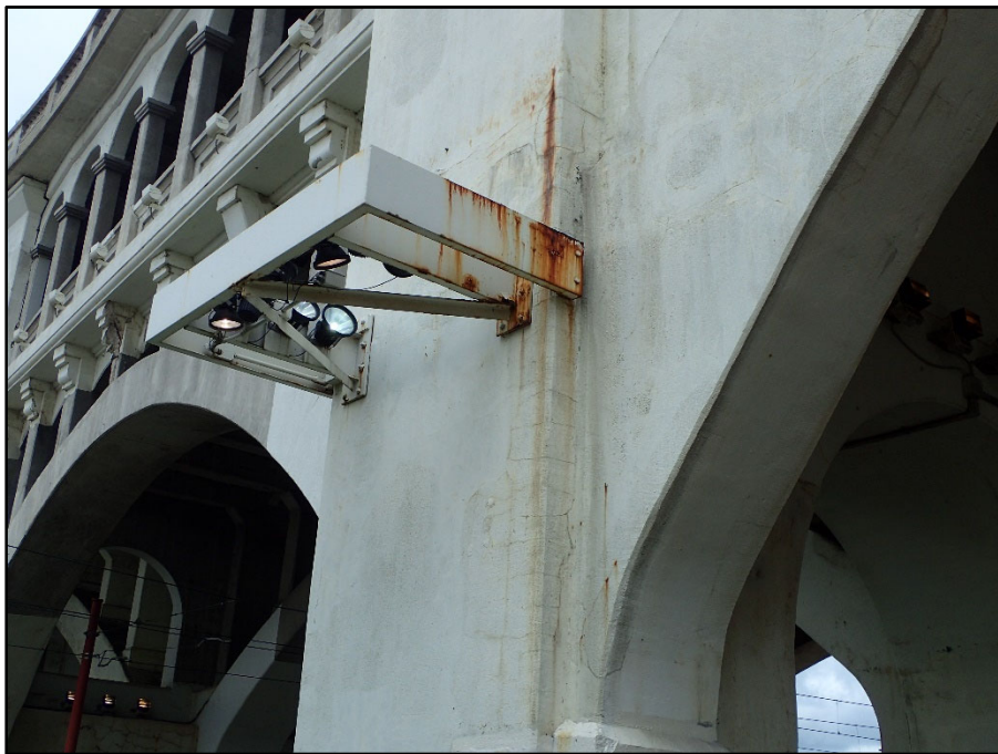
Photo 41 –Typical architectural lighting brackets on pier are corroding
