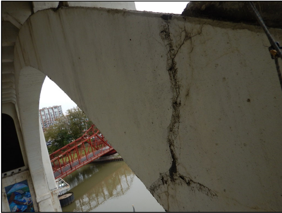
Photo 18 – Span 5 North Exterior Arch Rib, Panel 14; longitudinal through crack that has propagated into several spandrel columns
