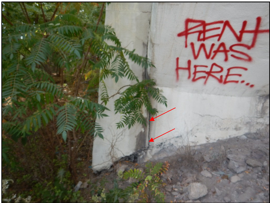
Photo 39 – West Abutment Below South Exterior Arch; 1/4" W vertical crack
