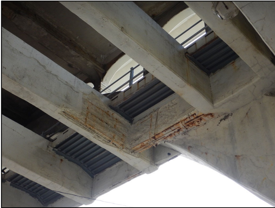
Photo 24 – Span 12, lower deck floorbeams; multiple floorbeams have spalled concrete with exposed, painted over reinforcing
