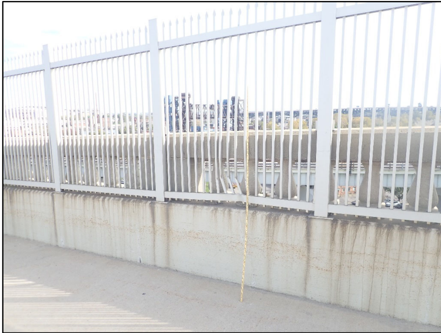
Photo 5 – Typical bridge rail condition
