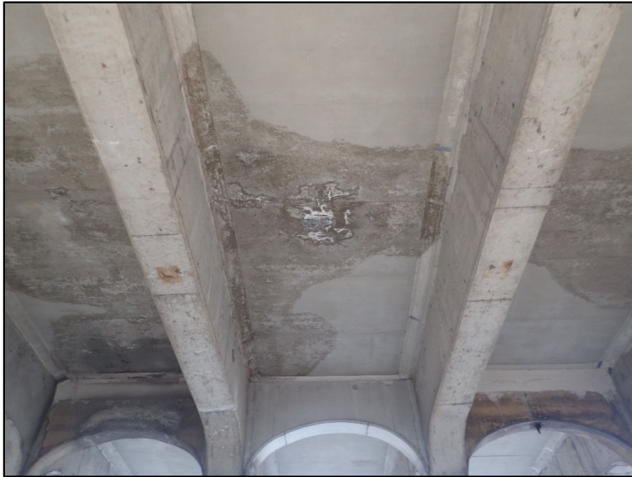
Photo 15 – Upper Deck, Span 7, Panel 4 center bay; local area of efflorescence
