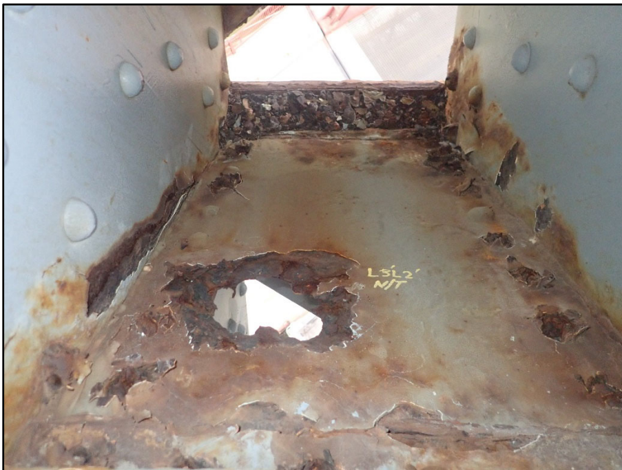
Photo 33 – Span 4 North Truss L3'L2' diaphragm; corrosion hole
