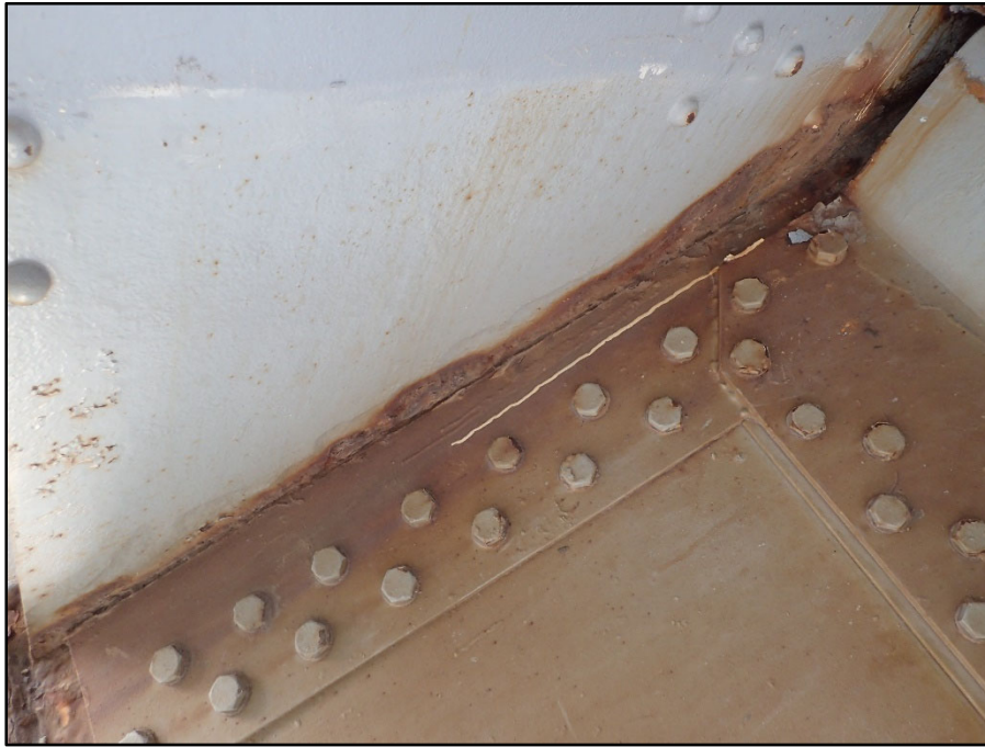
Photo 30 – Span 4 North Truss L3 south gusset above L2L3; Active laminar corrosion and pitting up to 3/16" D
