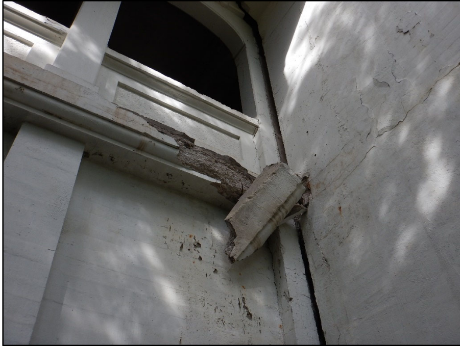
Photo 42 – Tower B South side; rotated outwards and fractured at the interface with the upper deck
