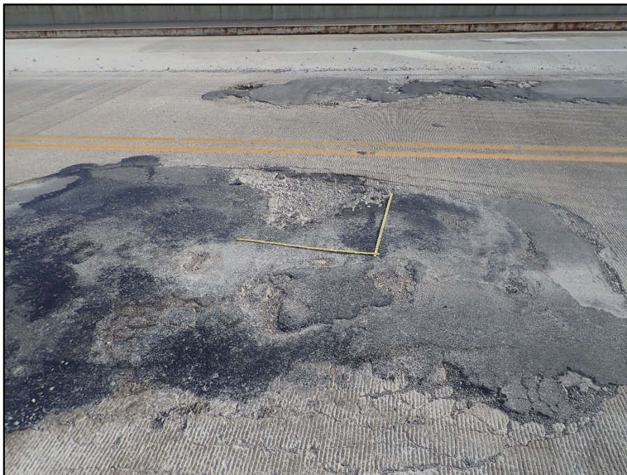
Photo 16 – Span 8 eastbound lane; 25' L x 7' W x up to 3" D spalling patch with exposed reinforcing
