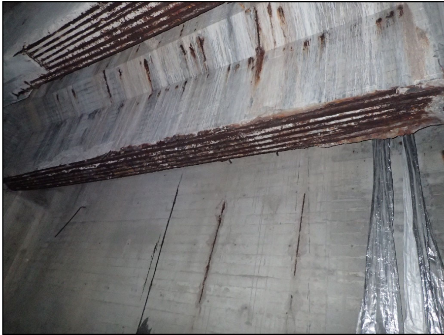
Photo 50 – East Abutment, North Chamber ceiling; bottom of floor beam spalled full length with exposed reinforcing
