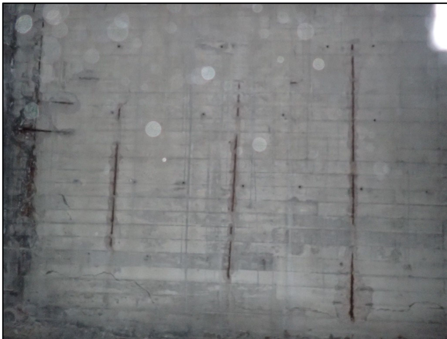
Photo 51 – East Abutment, South Chamber, west wall; vertical spalls with exposed reinforcing
