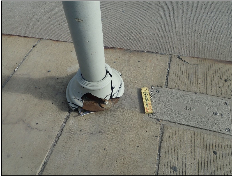
Photo 17 – Span 11, north sidewalk; broken light pole base
