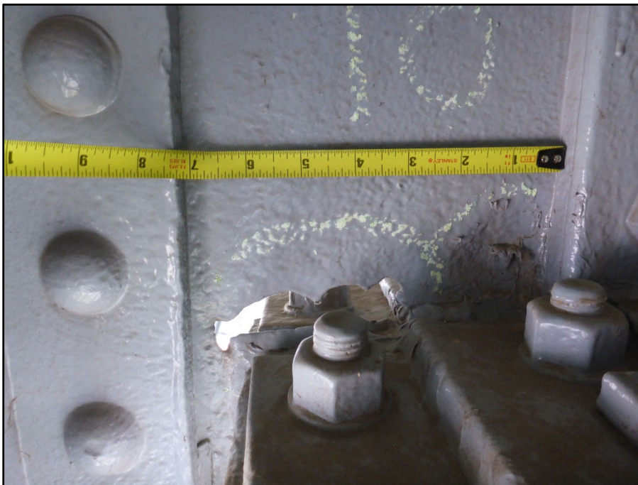
Photo 31 – Span 4 Upper Deck Floorbeam 10'; web corrosion hole north of the first interior stringer from the panel point
