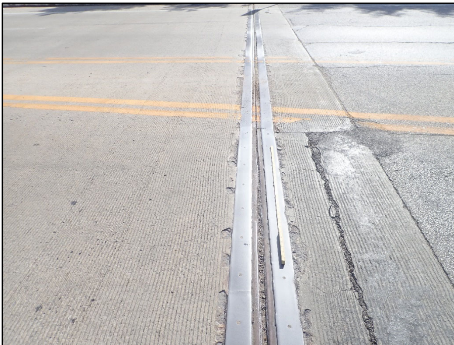
Photo 10 – Tower B expansion joint, left westbound lane; pack rust has broken fillet welds. Snow plow damage is present.
