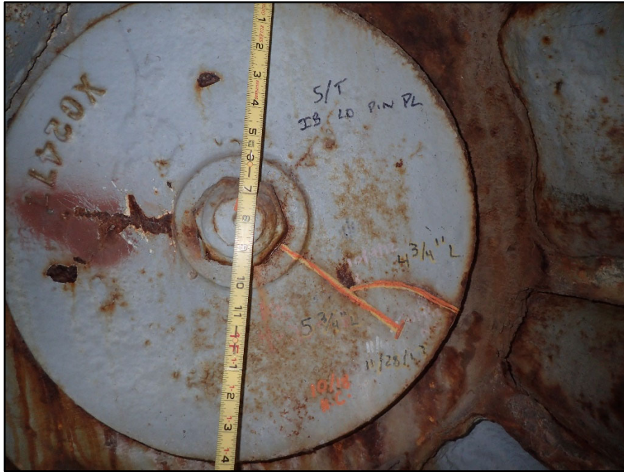
Photo 34 – Span 4 South Truss L0 Inboard Pin Cover Plate; non-structural plate with two cracks
