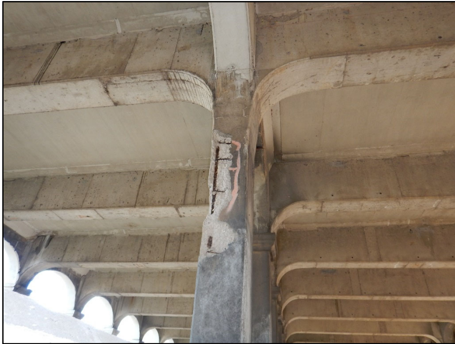
Photo 22 – Span 8 North Interior Upper Column 2; 4' H x 4" D corner spall on the northeast corner of the column with exposed reinforcing
