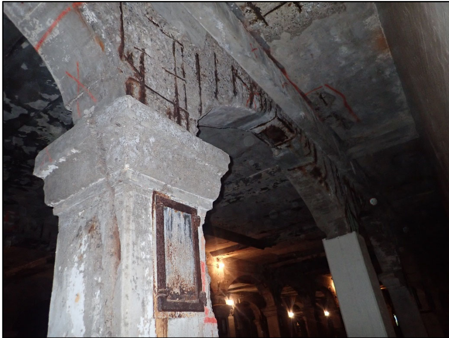
Photo 38 – West 25 th Street Columns and Arches; heavily deteriorated with exposed reinforcing and efflorescence
