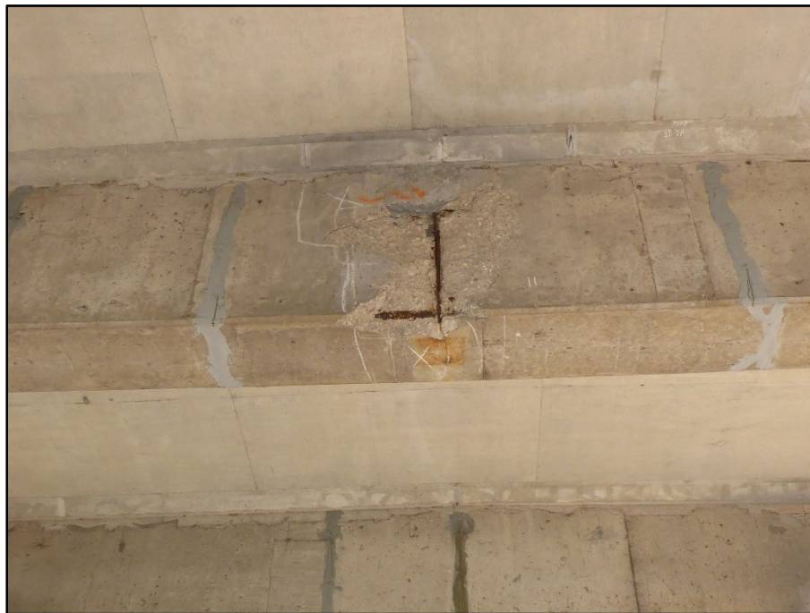
Photo 23 – Span 5 Upper Deck Floorbeam 11 west face between interior arches; Full Height x 3' W x 4" D spall with exposed rebar
