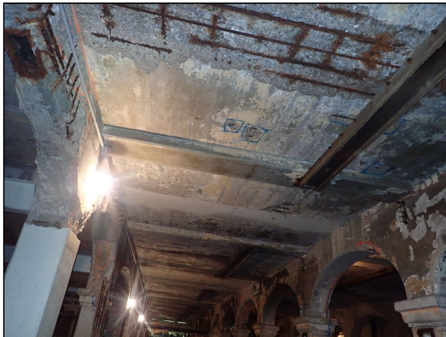
Photo 8 – West tunnels upper deck with heavy efflorescence, cracking, delaminations, and spalls with corroded reinforcing steel
