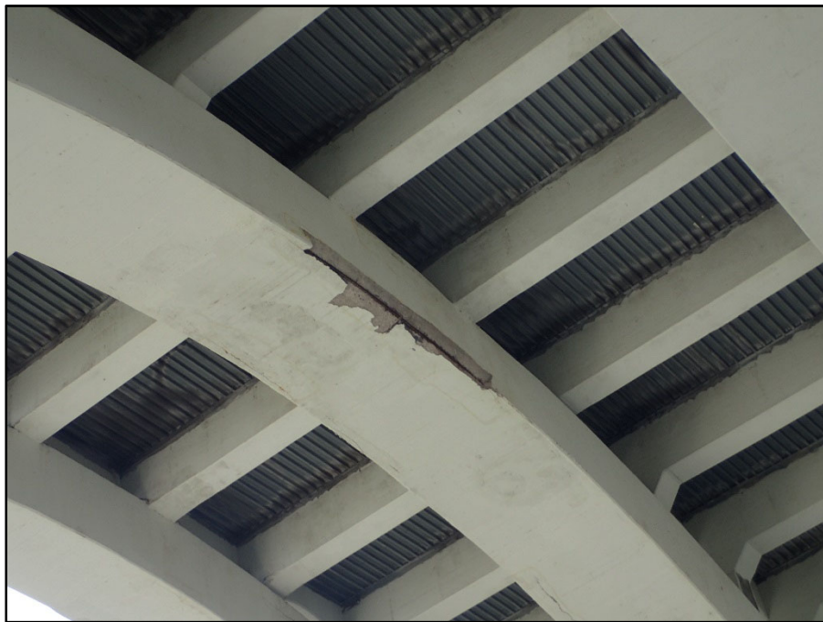
Photo 19 – Span 7 South Interior Arch Rib; lower north corner near apex has an unrepaired spall with exposed reinforcing
