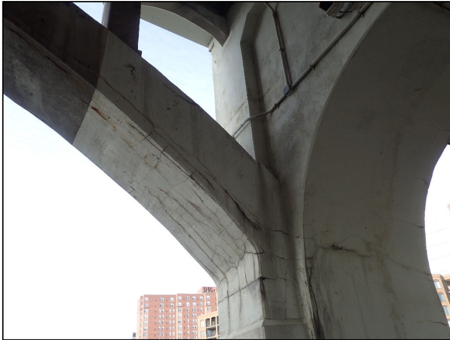
Photo 20 – Span 11 North Exterior Arch, south face; crack extending from Pier 11 up 1/4 length of the arch
