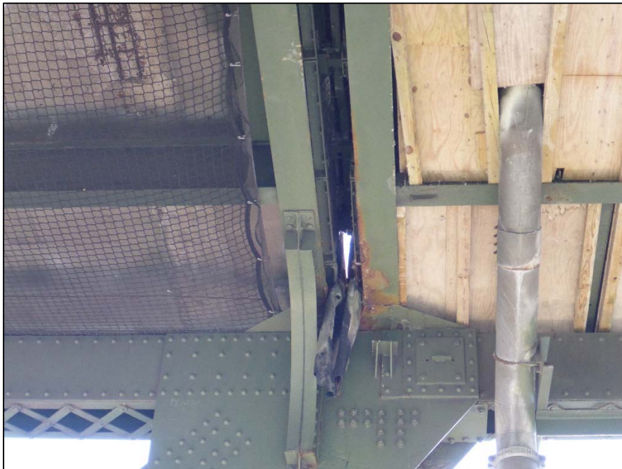
Photo 8 – Span 3 at panel point 13, South end of the joint; damaged/deboned with hanging material
