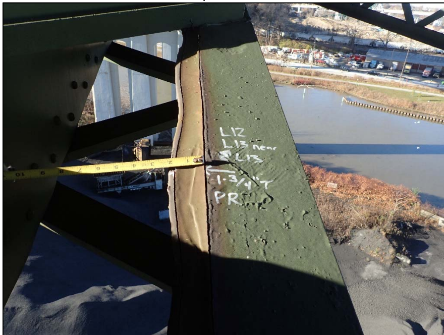
Photo 14 - Span 9 Interior lower chords; Up to 2" T pack rust between the upper flange angles
