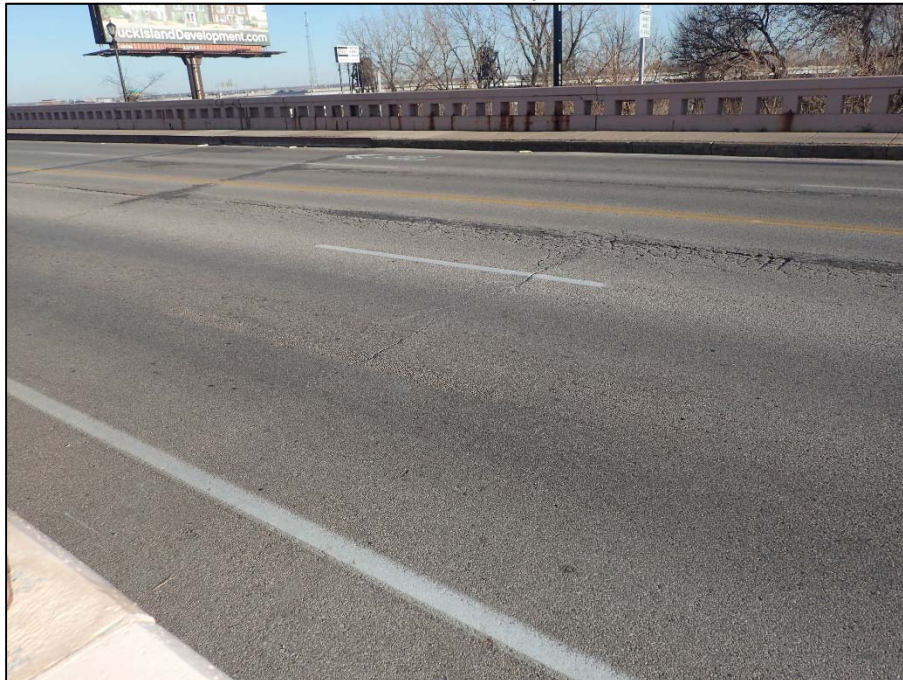
Photo 31 – West approach pavement has spalling, cracking and bituminous patching over 20% of the pavement
