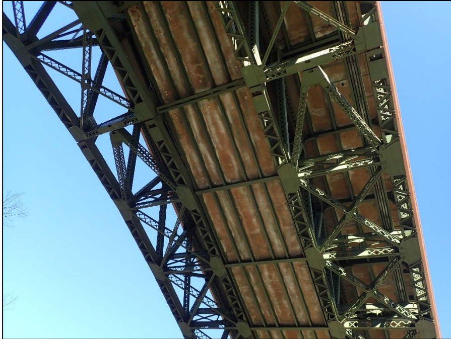
Photo 9 – Typical superstructure condition
