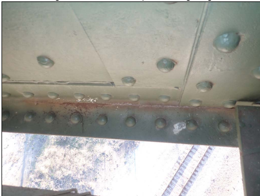
Photo 16 - Span 12, South Interior Truss at L3; Possible 35" L crack in the bottom North flange angle
