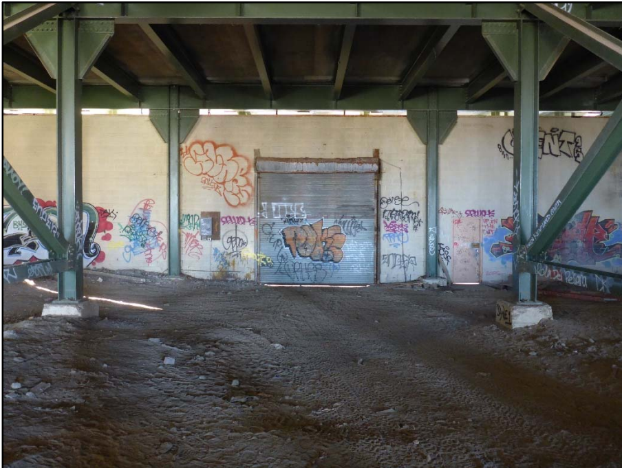
Photo 22 – West Abutment typical condition
