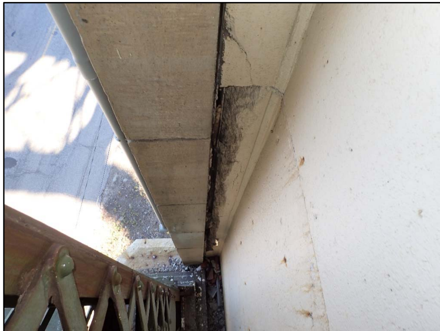
Photo 24 – East pylon backwall has a 12' H x up to 12" W spall/delamination behind the North Exterior Truss
