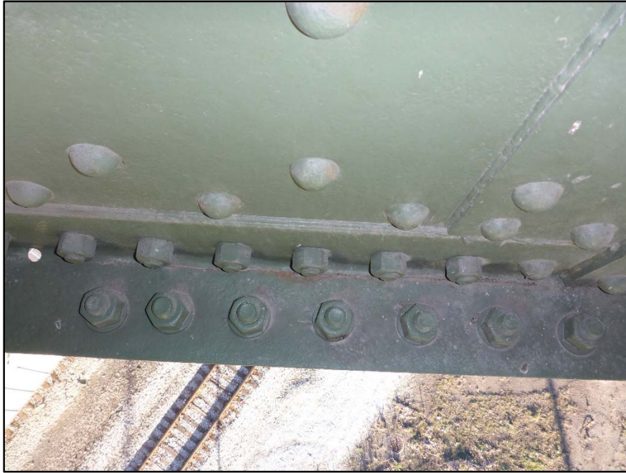
Photo 17 – Span 12, North Interior Truss at L4; Approximately 30" L crack with an arrestor hole drilled at the West end in the bottom South flange angle.
