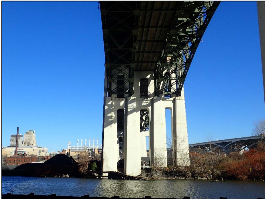
Photo 26 – Pier 9 bulkhead has failed along the East bank
