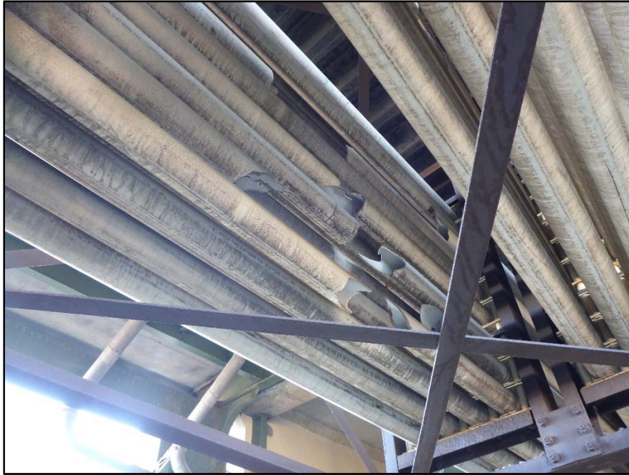
Photo 29 – Span 13, damaged area of conduit
