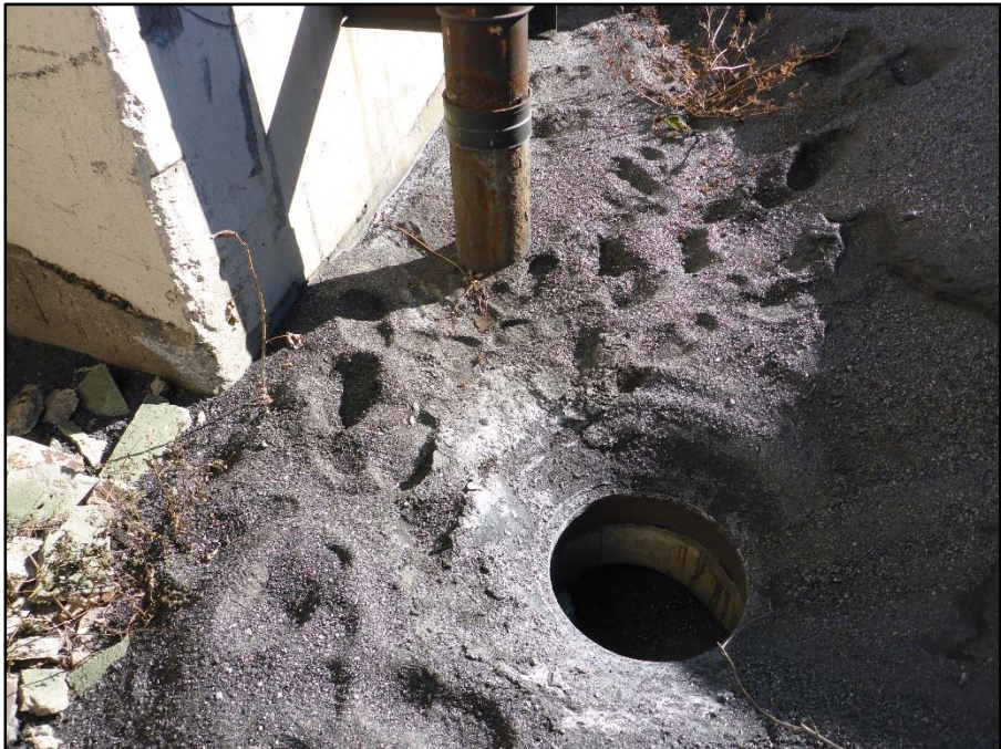
Photo 32 – Embankment on West face of Pier 6 has an open manhole
