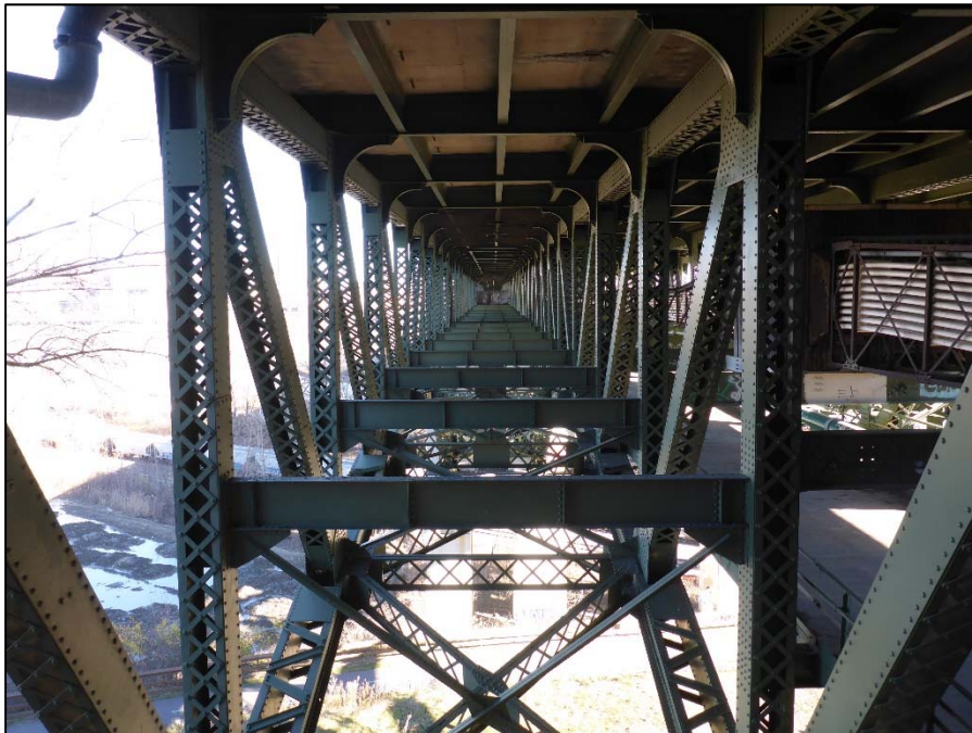
Photo 10 – Typical truss condition
