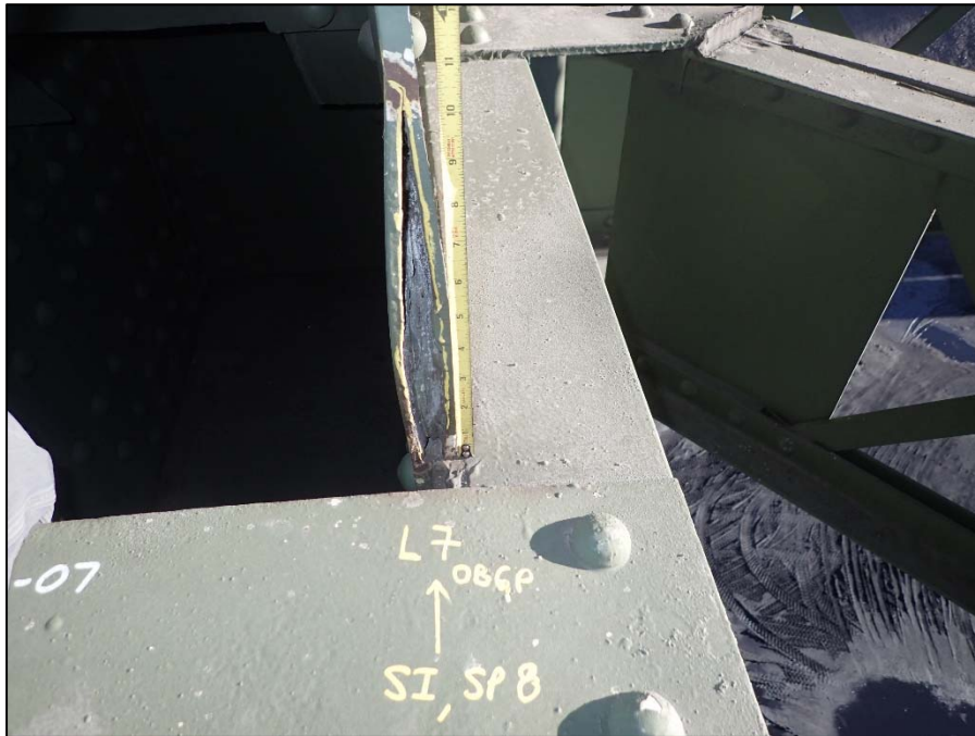
Photo 13 - South Interior Truss, L7; South lower chord gusset plate has a 10-1/2" H x up to 1" W laminar tear
