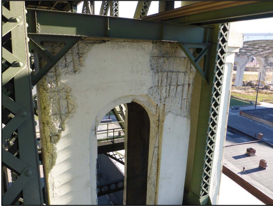
Photo 25 – West faces of Pier 4 have large painted over spalls with exposed reinforcing along the top behind the South truss line
