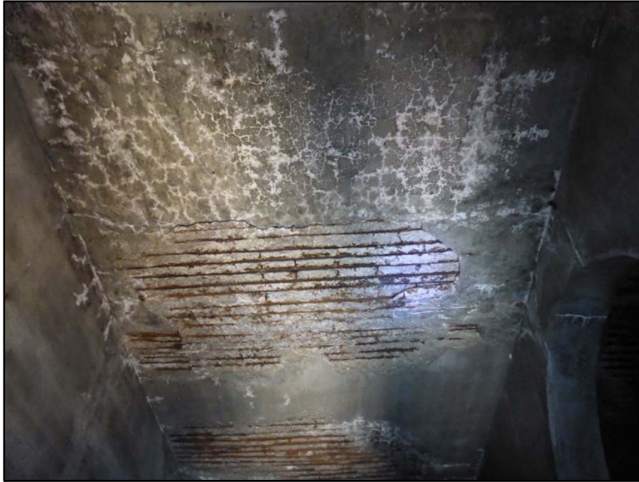
Photo 30 – East approach tunnel has large spalled areas with exposed rebar in all bays
