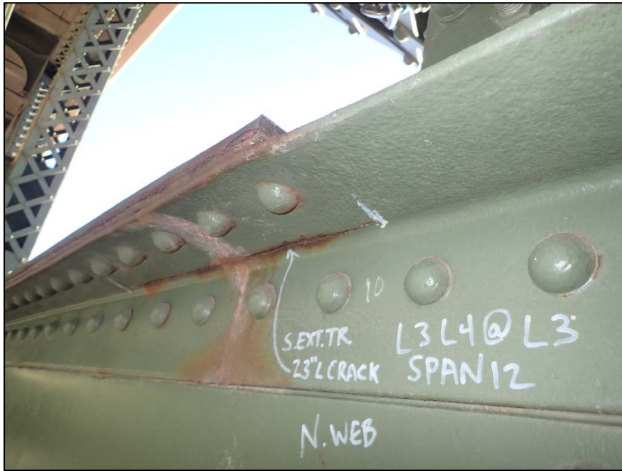
Photo 15 - Span 12, South Exterior Truss L3-L4 at L3; 23" L longitudinal crack in the top North flange angle
