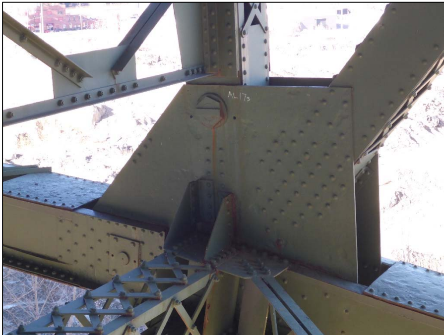
Photo 12 – Typical paint condition at panel points
