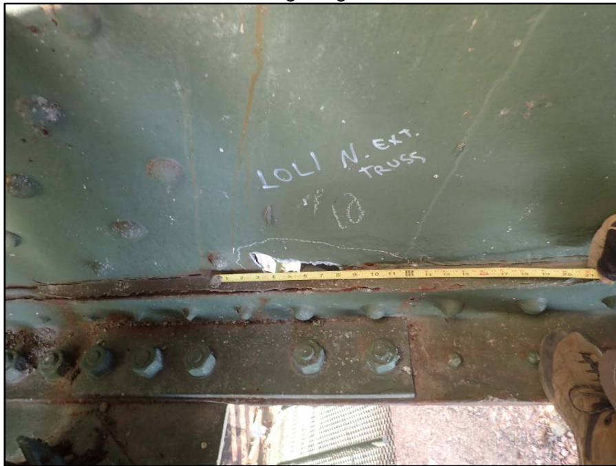
Photo 18 – Span 13; Typical lower chord section loss with perforations
