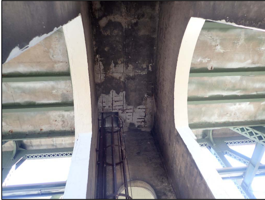
Photo 23 – Underside of Pier 12 cap, Typical condition
