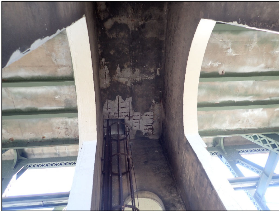
Photo 29 – Underside of Pier 12 cap, Typical condition
