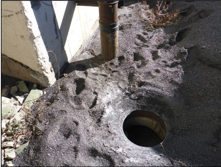
Photo 38 – Embankment on West face of Pier 6 has an open manhole
