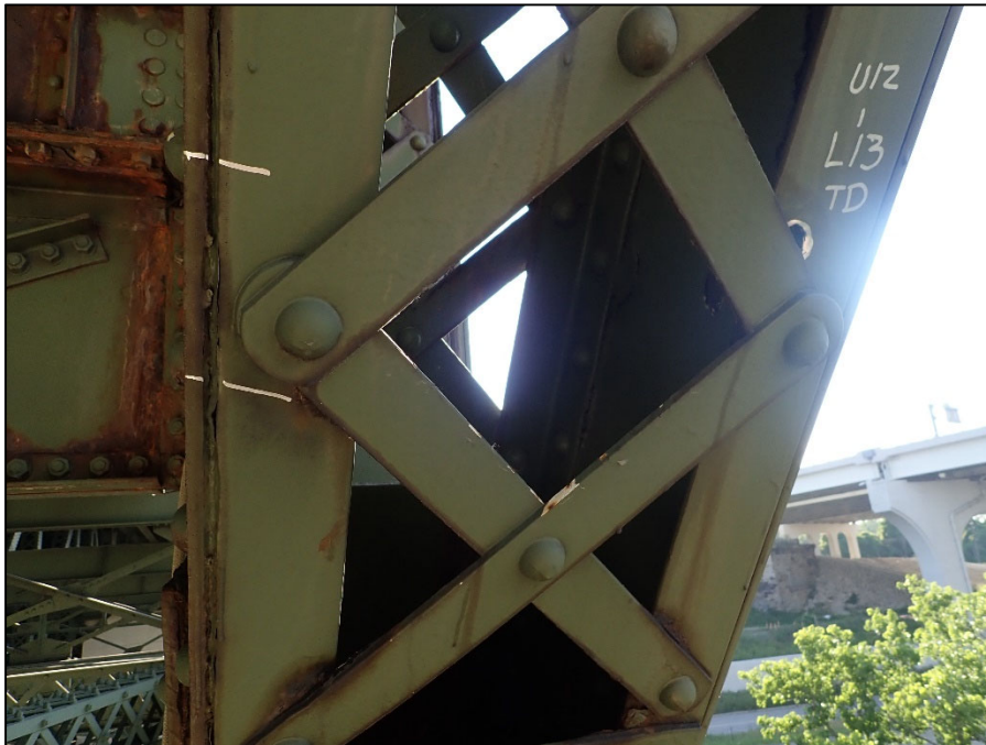
Photo 14 - South Exterior Truss, Span 3, U12L13; pack rust and corrosion holes
