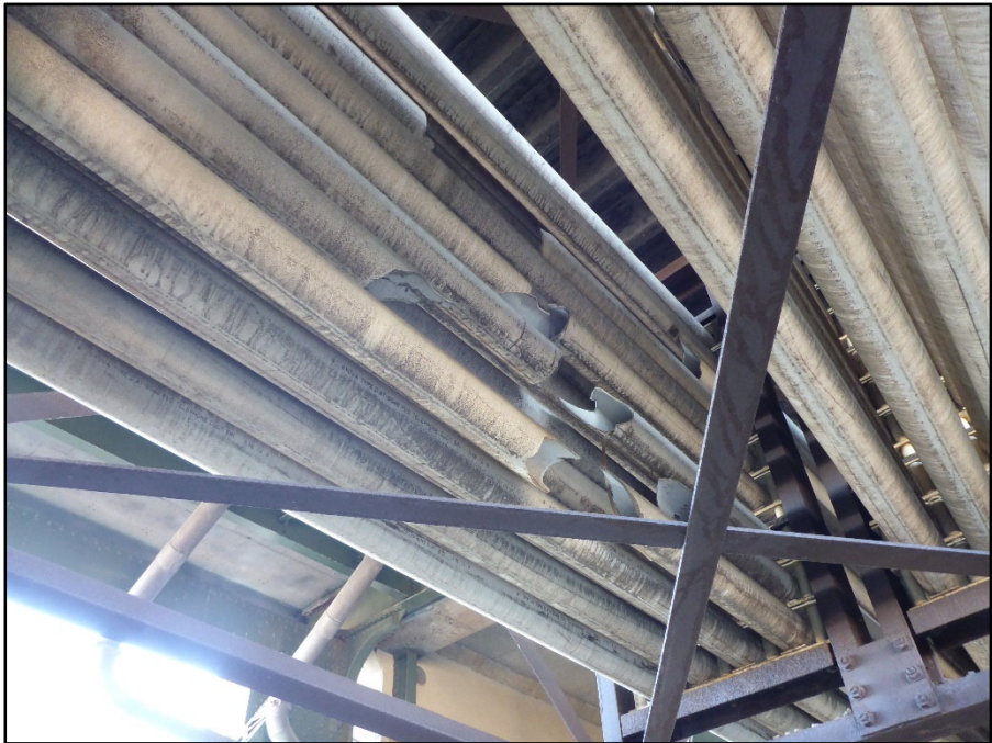
Photo 35 – Span 13, damaged area of conduit
