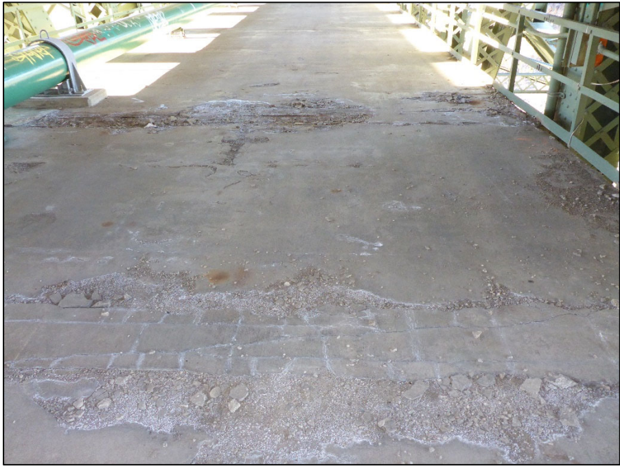
Photo 4 – Typical lower deck wearing surface; Cracking and delaminations with isolated spalling
