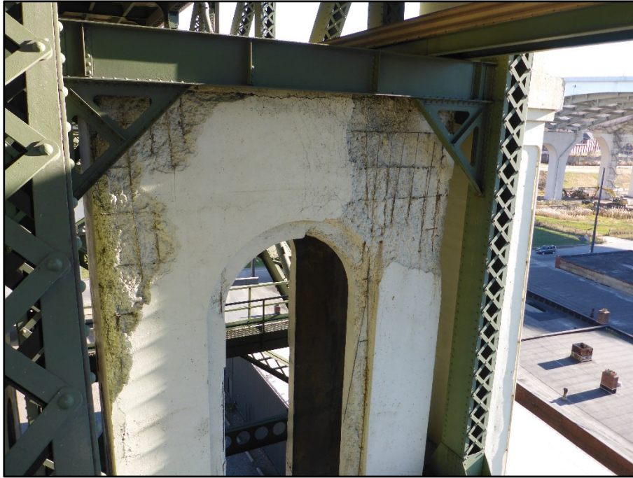
Photo 31 – West faces of Pier 4 have large painted over spalls with exposed reinforcing along the top behind the South truss line
