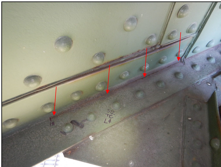
Photo 18 – South Interior truss, Span 12, L3L4; south lower angle at L4 with a 38-1/4" L crack
