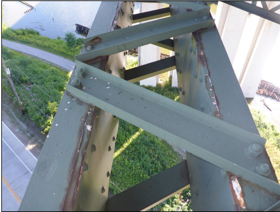
Photo 15 – North Exterior Truss, Span 11, L8L9; typical pack rust between lower chord built up members
