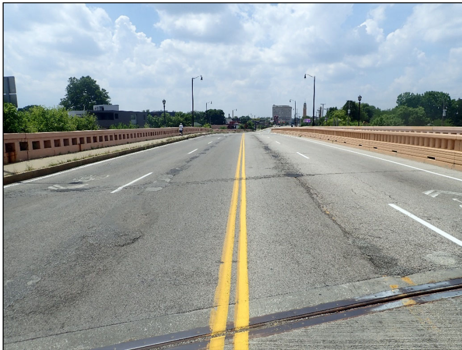
Photo 37 – West approach pavement has spalling, cracking, and bituminous patching over 20% of the pavement
