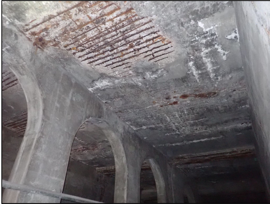
Photo 36 – East approach tunnel has large spalled areas with exposed rebar in all bays
