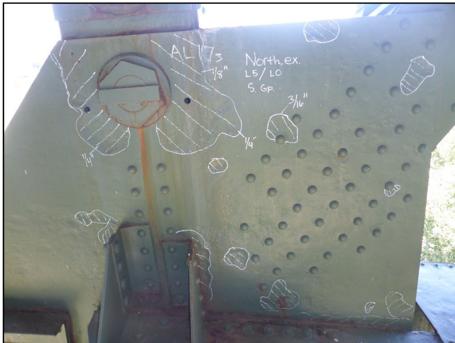
Photo 20 – North Exterior Truss, Span 11, L0 south Gusset Plate; Typical painted over pitting up to 1/4" D
