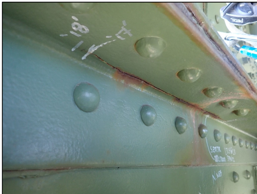
Photo 24 –South Exterior truss Span 12, L3; 23-3/4" L longitudinal crack in inboard top north flange angle (3/4" growth since previous inspection)
