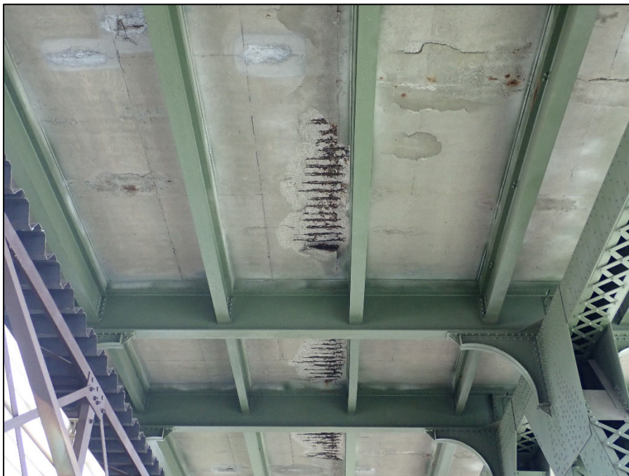
Photo 2 - Typical underside of deck spalling with exposed rebar and delaminations
