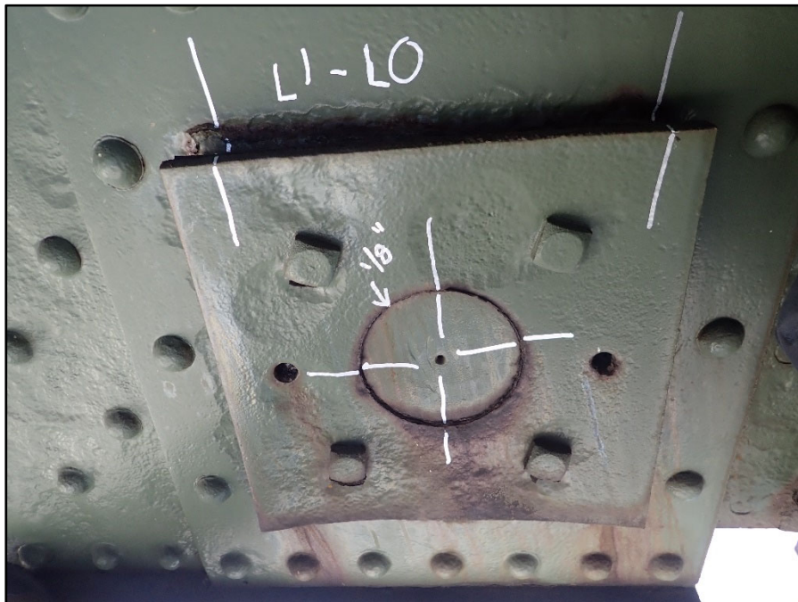
Photo 22 – South Exterior Truss, Span 8, L0; Typical corrosion and pack rust around pin and plate
