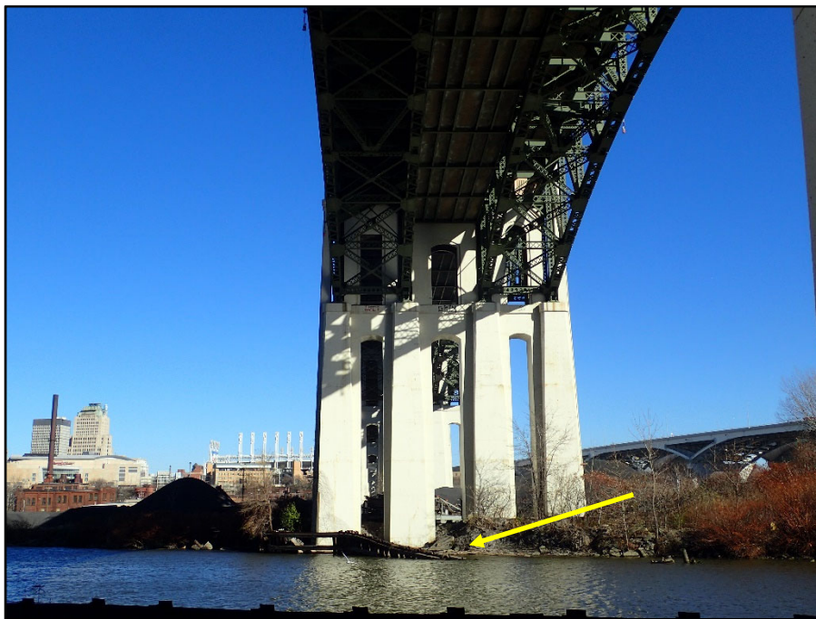
Photo 32 – Pier 9 bulkhead has failed along the East bank
