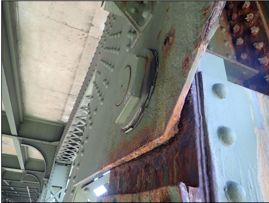
Photo 13 - South Interior Truss, Span 7, L15U15 at U15; Vertical below deck joint with active corrosion and pack rust
