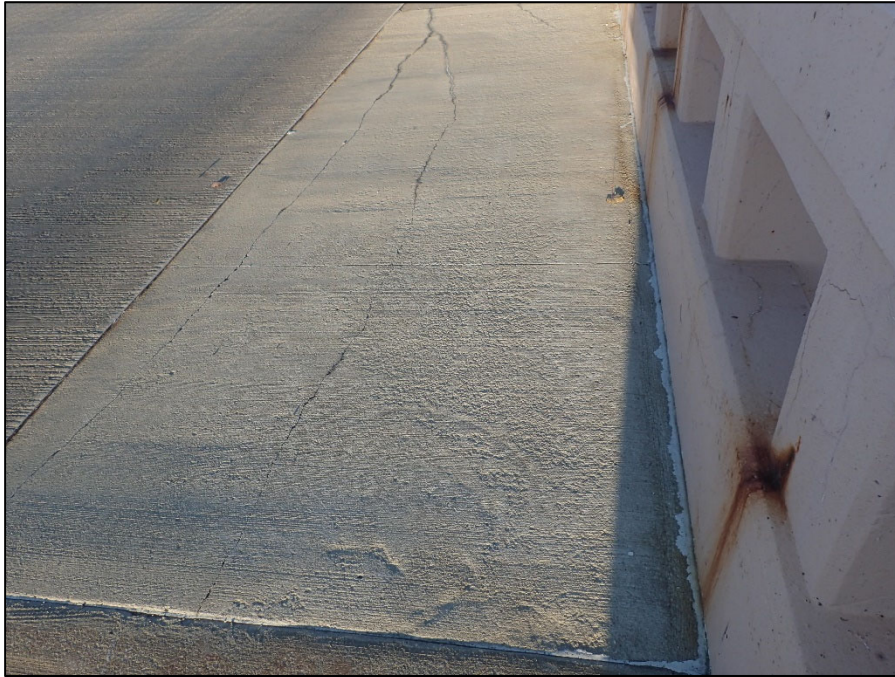
Photo 5 - South sidewalk; 18' L x up to 1/4" W longitudinal crack with associated minor edge spalling
