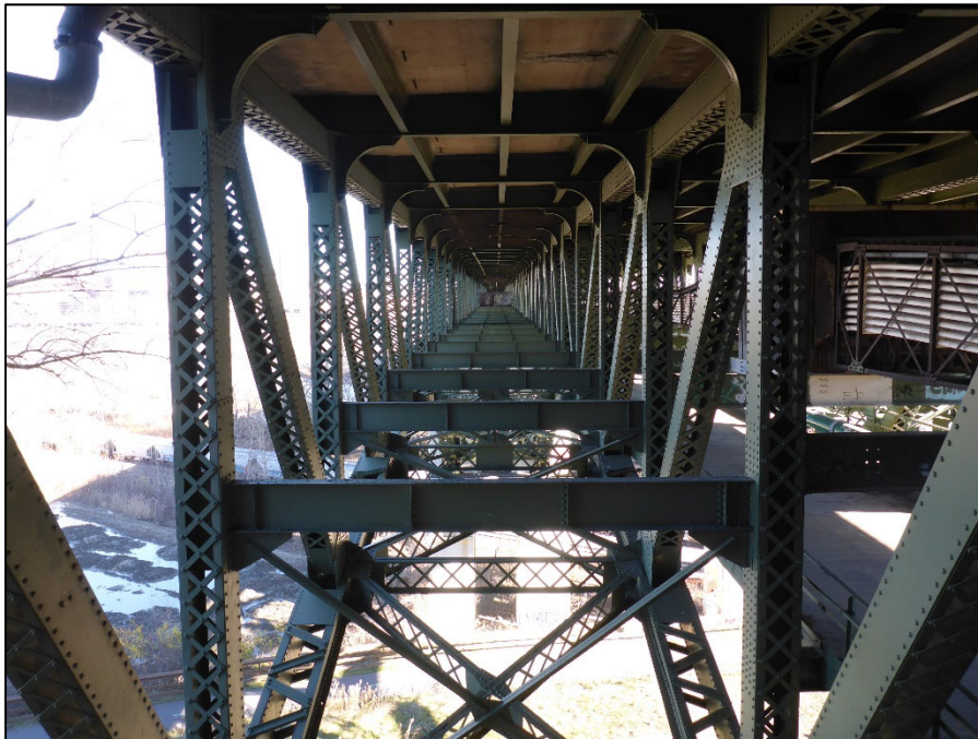
Photo 10 – Typical truss condition
