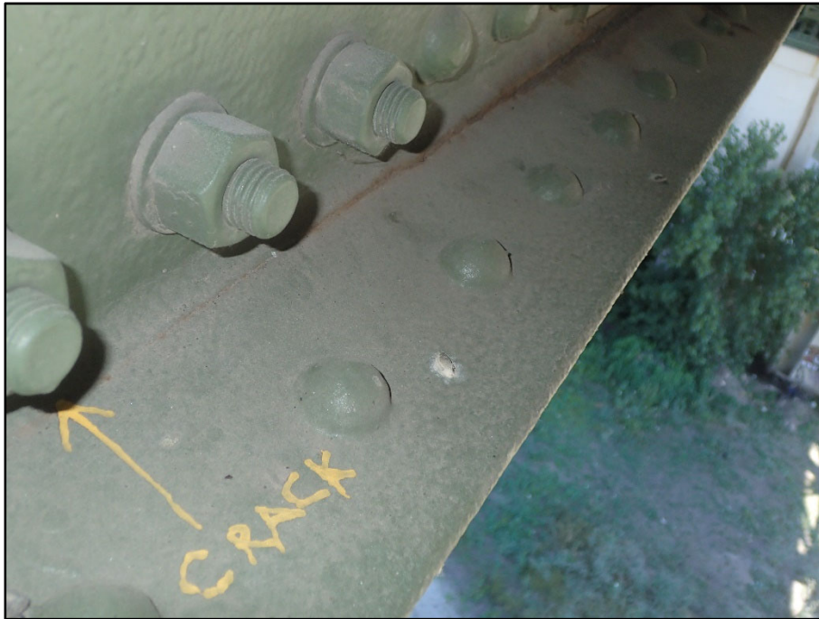
Photo 17 – North Interior Truss, Span 12, L1L2; 6'-4" L crack with an arrestor hole at the east end of crack
