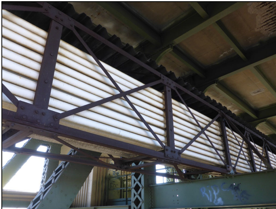
Photo 34 – Typical Telecom conduits
