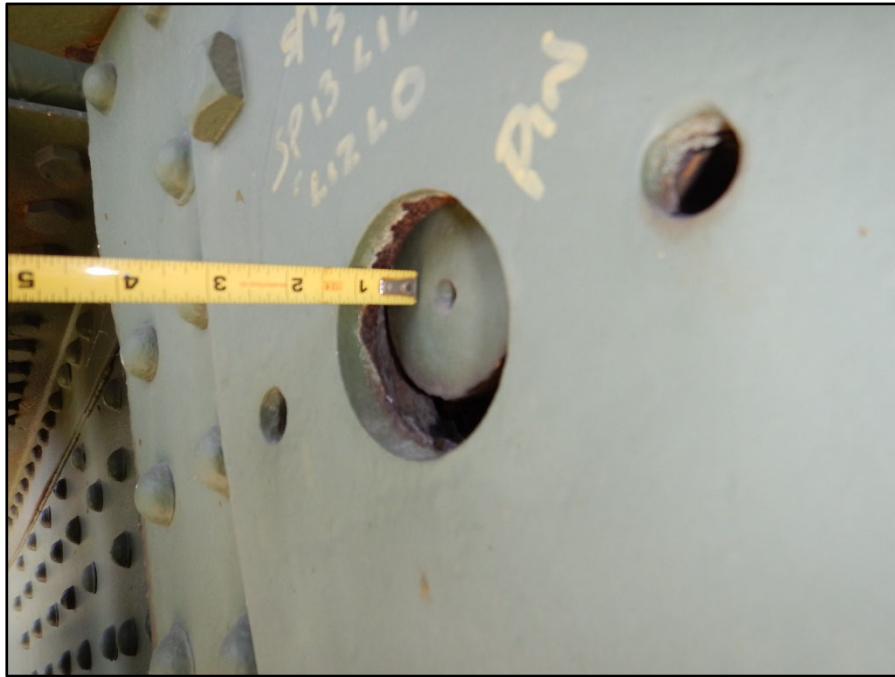
Photo 23 – South Interior Truss, Span 12, L0; dislodged pin
