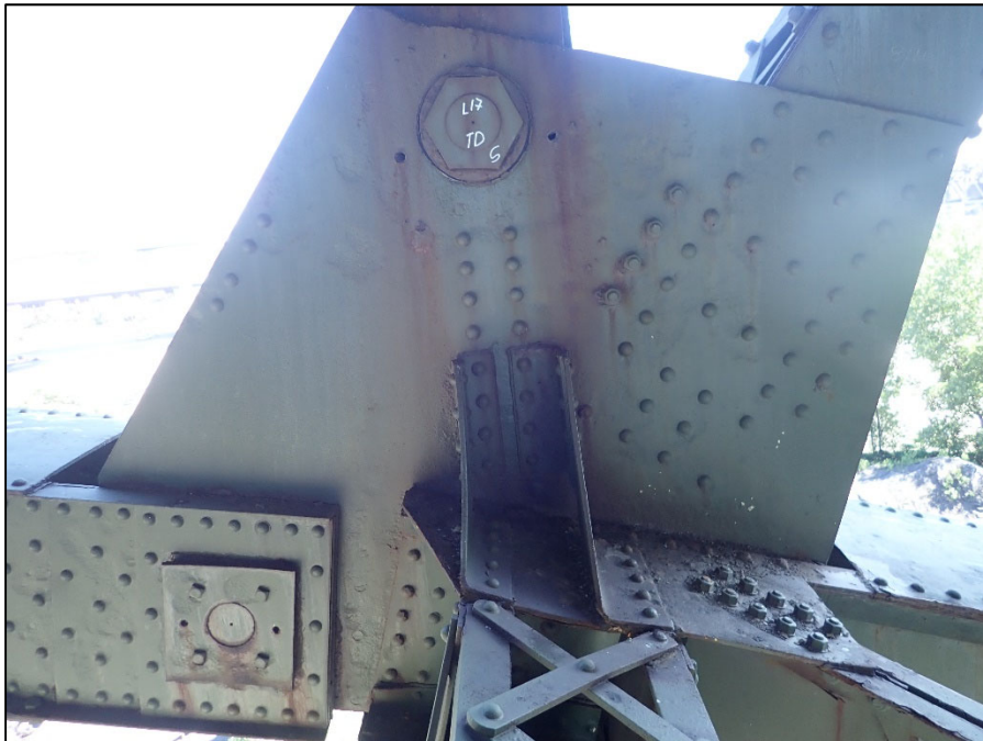
Photo 12 – Typical paint condition at panel points
