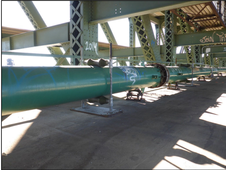
Photo 33 – Typical gas line on lower deck
