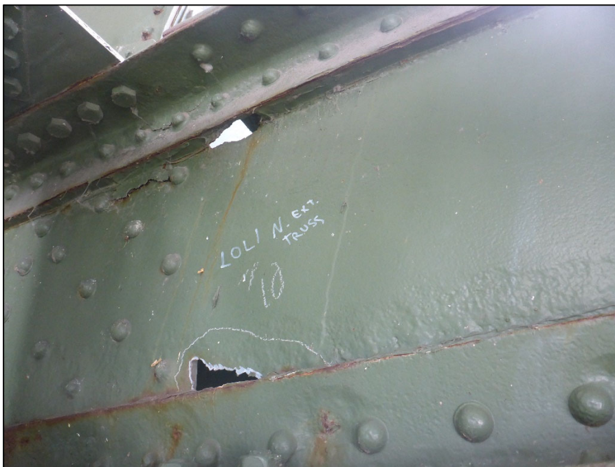
Photo 16 – North Exterior Truss, Span 13, L0L1; corrosion holes in lower chord web
