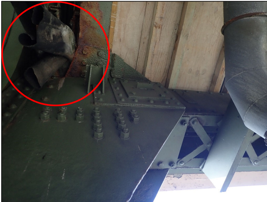
Photo 8 – Span 3 at panel point 13, South end of the joint; damaged/de-bonded with hanging material
