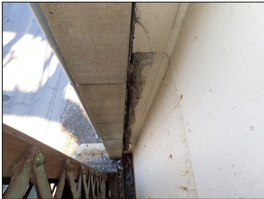
Photo 30 – East pylon backwall has a 12' H x up to 12" W spall/delamination behind the North Exterior Truss
