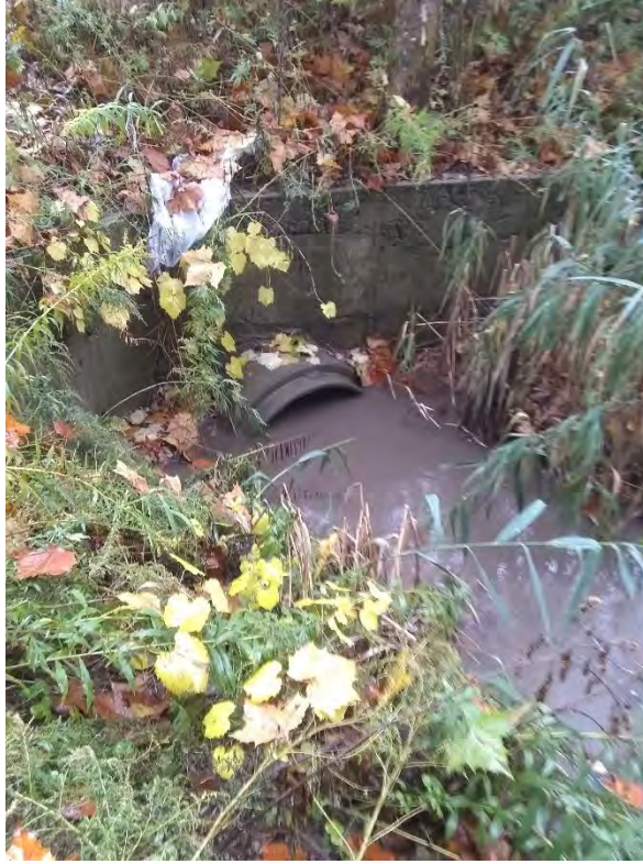
Photo 27. PIP 16 – 10/29/20 – Suspended Solids in Water, No Odor
