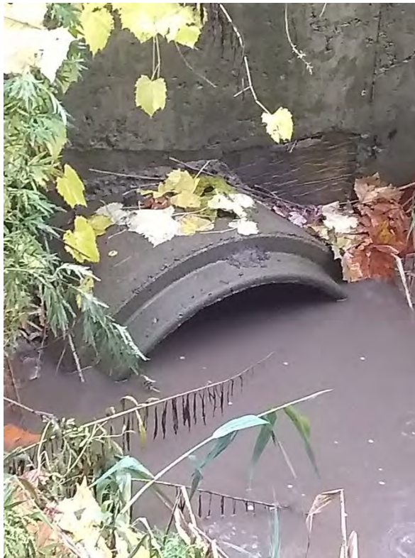
Photo 28. PIP 16 – 10/29/20 – Suspended Solids in Water, No Odor
