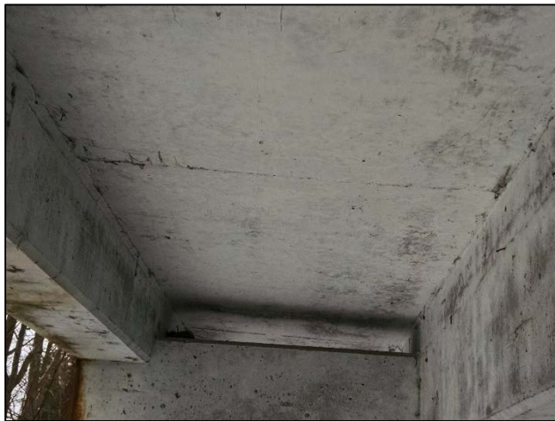
Photo 7 – Typical good condition of the bottom of the sidewalk slab. West Approach, South sidewalk shown.
