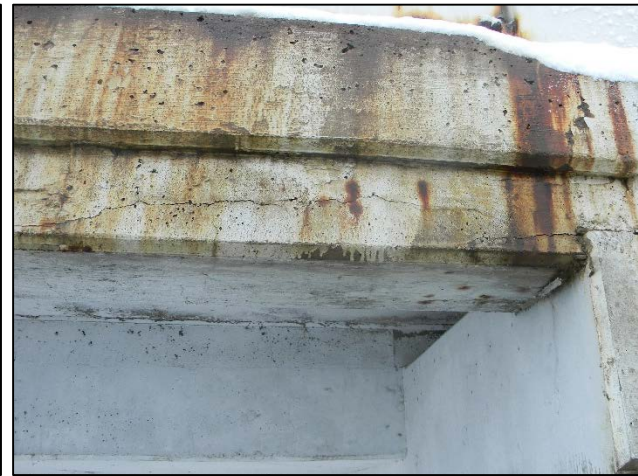
Photo 2 – Typical longitudinal cracks along the vertical face of the sidewalk fascia beam. North Sidewalk, Arch H Bay 4 Shown.
