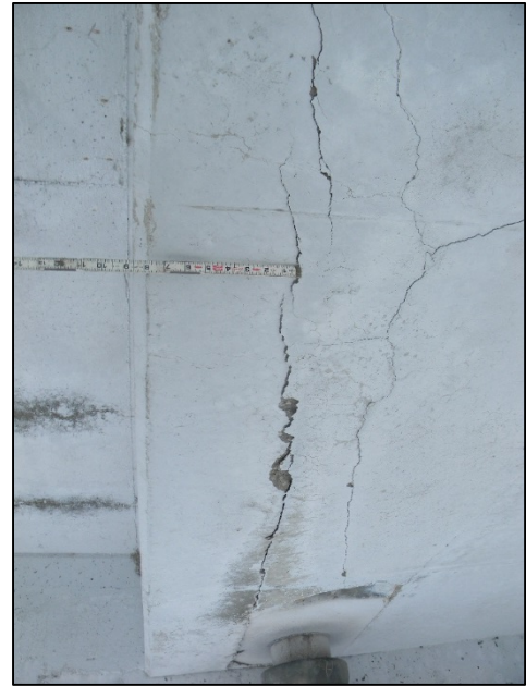
Photo 6 – Large delaminated area beginning approximately 9" from the back of the curb beam, approximately 12" by 4 feet. North Sidewalk, Arch D Bay 1 shown.
