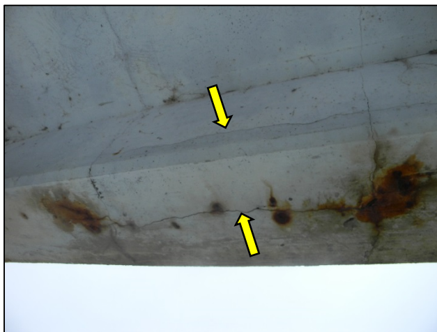
Photo 3 – Typical corner delamination with side and bottom cracks pointed out. North Sidewalk, Arch E Bay 5 shown.
