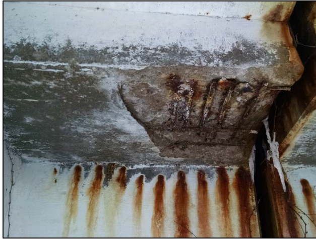
Photo 5 – Curb beam and deck soffit delaminated and spalled to bottom mat at the West Pylon joint. South Sidewalk shown.
