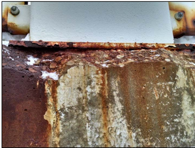
Photo 1 – Top Corner spall exposing approximately 1/4" of bottom of post base plate. Fourth post of Arch B, South Sidewalk shown.
