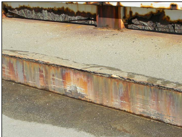
Photo 8 – Portion of an 11 foot long, 1 foot wide delamination of the Arch B North sidewalk. Water and rust is buckling the delaminated layer of concrete up.
