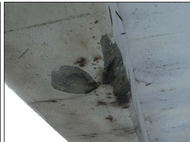
Photo 4 – Typical corner spalling along the fascia beam bottom. 2"x2"x9" spall and 3" diameter spall shown at North Sidewalk, Arch D Bay 2.
