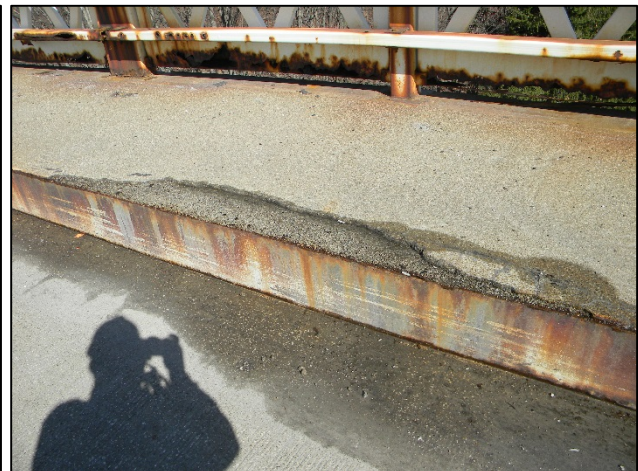
Photo 9 – Another Arch B North sidewalk location showing asphalt fill in a spalled portion of the sidewalk.
