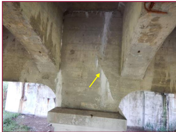
Vertical hairline crack with moderate efflorescence on the west face of the diaphragm between Beams 5 & 6 at Pier 14 (looking east).
