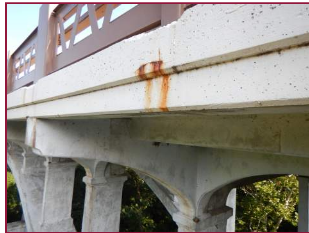
Typical longitudinal and transverse hairline cracks in the sidewalks (looking southeast).
