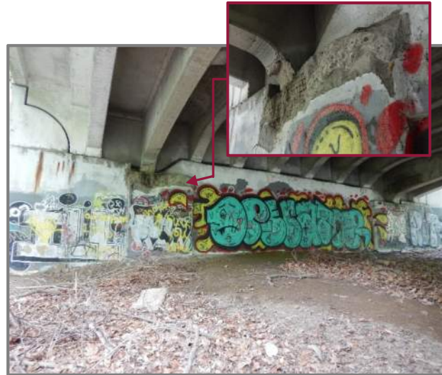
Photo 32 – East elevation of the Rear Abutment (looking west). Inset: Looking southwest at the spall with exposed reinforcement in the right relief.
