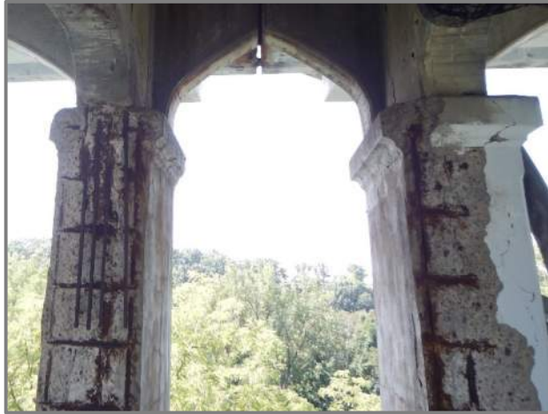
Photo 24 – Typical spalls with exposed reinforcement in the arch spandrel columns below the joints (looking south at right columns near Pier 9).
