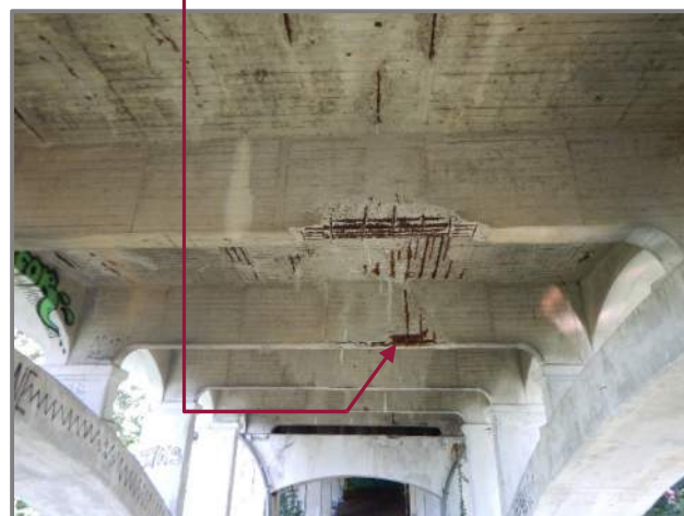
Photo 26 – Spalls with 3 broken stirrups in Floorbeams A3 and A4 (looking west). Inset: Looking northwest at Floorbeam A3 where a 10' long delamination was removed.
