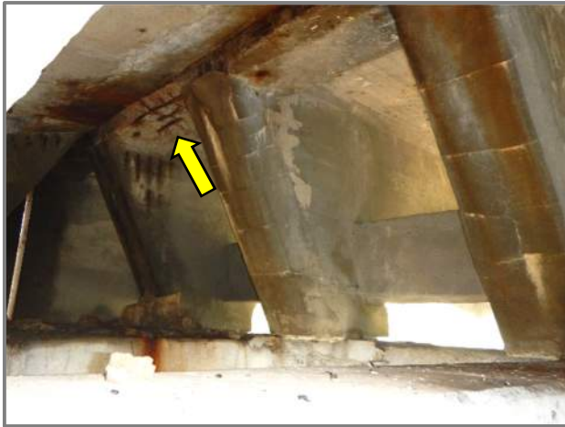
Photo 5 – Deck underside at the East Pylon with a large spall with exposed reinforcement between Beams 2 and 3 in Span 15 (looking northeast).
