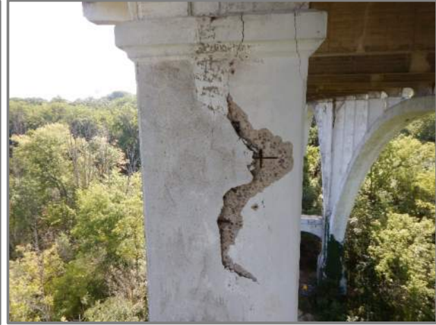
Photo 25 – Spall/delamination 8' high in the rear face of the Span D left arch Spandrel Column 2 (looking east).
