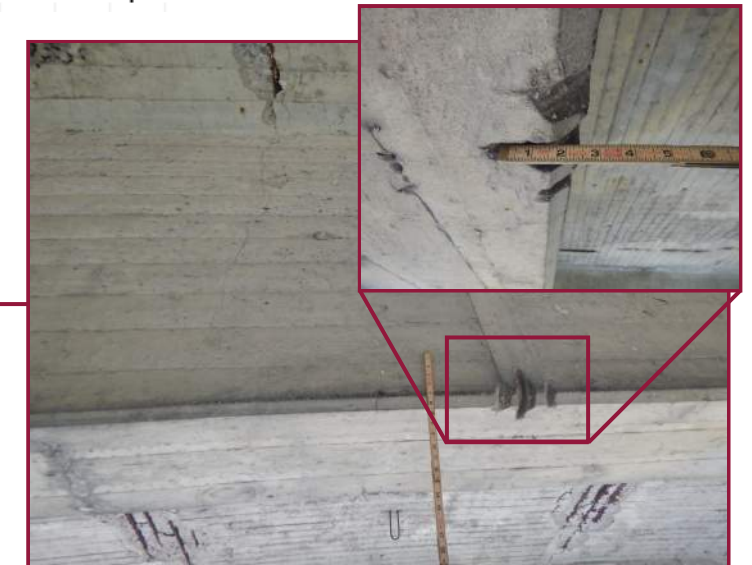
Gouges in the west face near the bottom of Floorbeam A7 near midpoint between the Left and Right Jack Arch (looking east).
