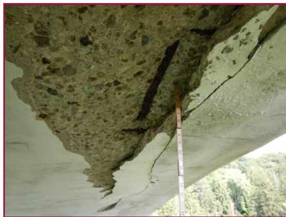
5' long by 2' wide by 4" deep spall on the bottom face of the North Arch between Spandrel Columns 4 & 5 (looking west).
