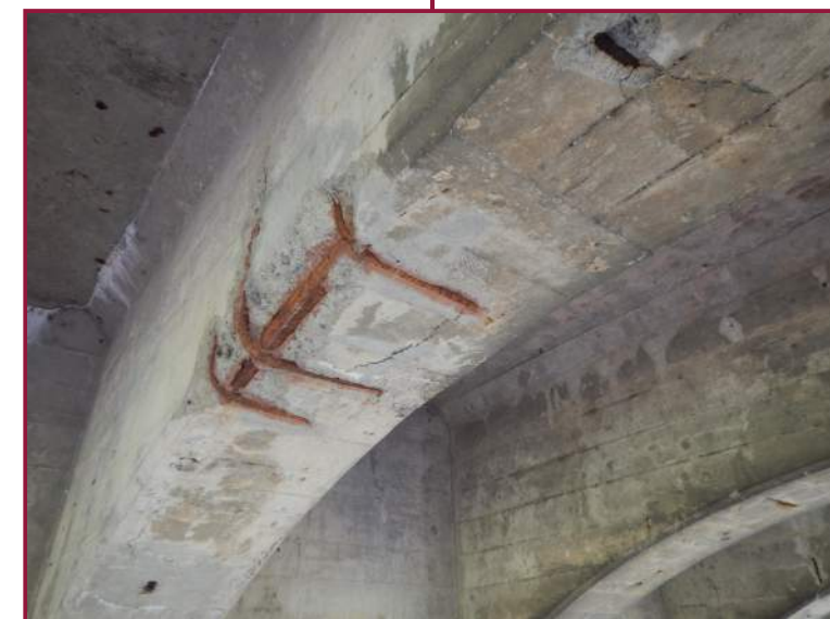
18" long by 12" wide spall with exposed reinforcement on the north face bottom edge of Beam 6 near Pier 14 (looking southeast).
