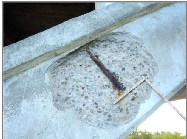
Photo 23 – Spall with exposed reinforcement where a delamination in the Span B left arch was safely removed during the inspection (looking south above the east shoulder of Valley Parkway and below Column 8).
