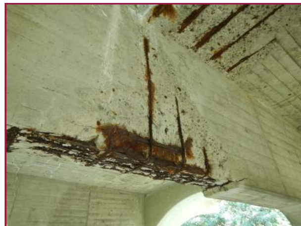
10" long by 4" high by 3" deep spall with exposed and broken reinforcement on the east and bottom face of Floorbeam A3 near midpoint between the Left and Right Jack Arch (looking west).
