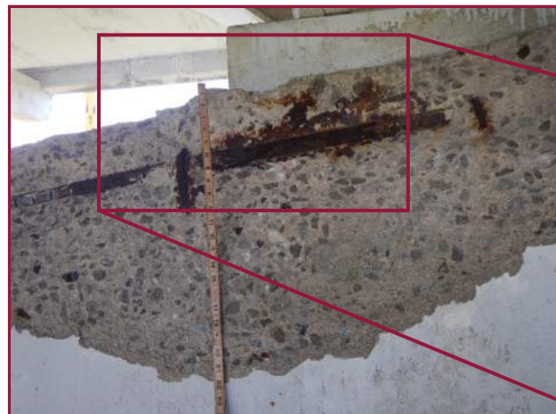
Top edge spall with exposed reinforcement on the north face of the South Arch below Column 6 (looking south).
