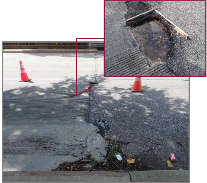
Photo 39 – Rear approach slab with a failed patch/pothole at the rear edge (looking west). Note the cracking along the rear edge of the slab.
