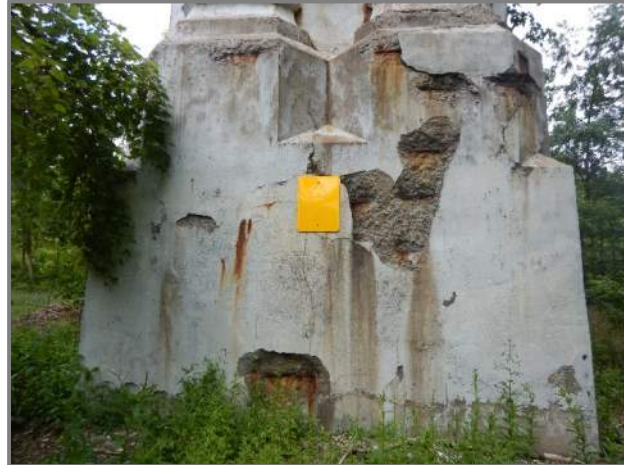
Photo 29 – Spalls with exposed reinforcement throughout the Pier 8 right column exterior face (looking north). Note the nearly fully faded falling concrete warning sign.
