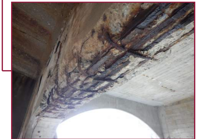
Spall with exposed reinforcement and nine stirrups with 100% section loss on the east face Pier 12 near the Right Jack Arch on the South Arch (looking west).
