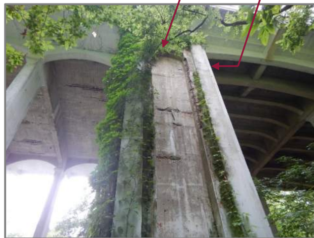
Photo 30 – West Pylon left column exterior face with spalls with exposed reinforcement and vegetation growth (looking south at the left face). Top left inset: Looking south. Top right inset: Looking east at the top of the column on the left side of Beam 1.
