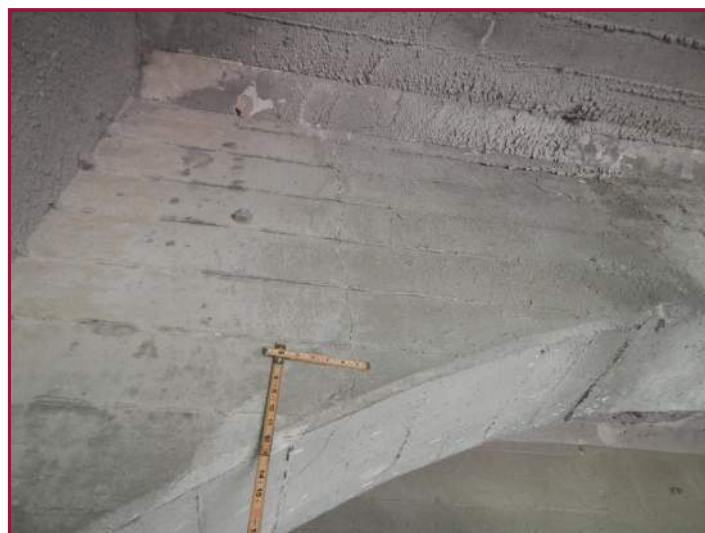
Full height vertical crack up to 1/16" wide at the east end of the Beam 4 north face (looking south).
