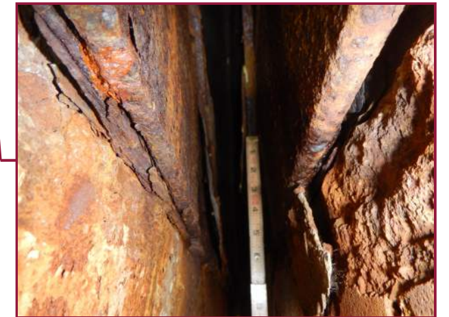
Up to 1/2" thick laminate corrosion throughout the interior face of the joint armor at Pier 7 at the Right Arch (looking north).
