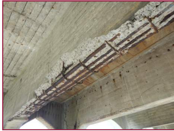
20' long by 18" high by full width spall with exposed reinforcement including 5 broken stirrups on the underside of Pier 10 (looking southwest).
