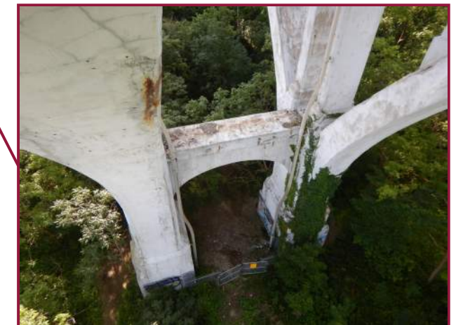
Vegetation growth on the west face of the south column of Pier 9 (looking southeast).
