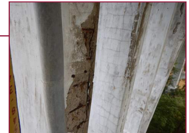
Full width by 6' high edge spall with exposed reinforcement on the south face of the North Spandrel Column at Pier 11 (looking northeast).
