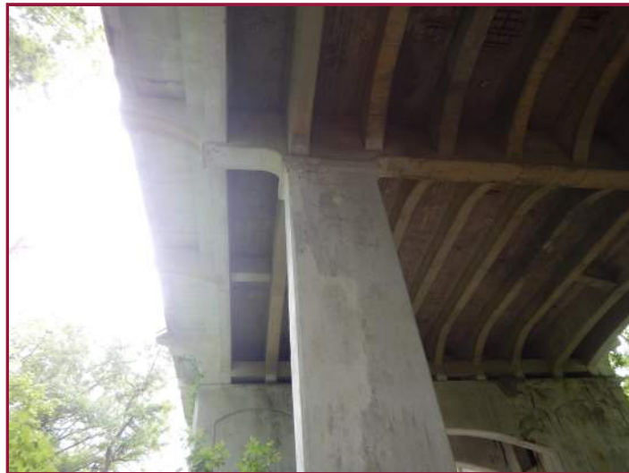
Hairline map cracking at a patch in the approach pier column (looking east).
