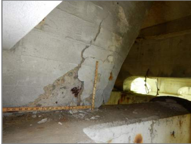
Photo 21 – Spall and delamination in the end of Beam 4 at the West Pylon (looking northeast in Span 6).
