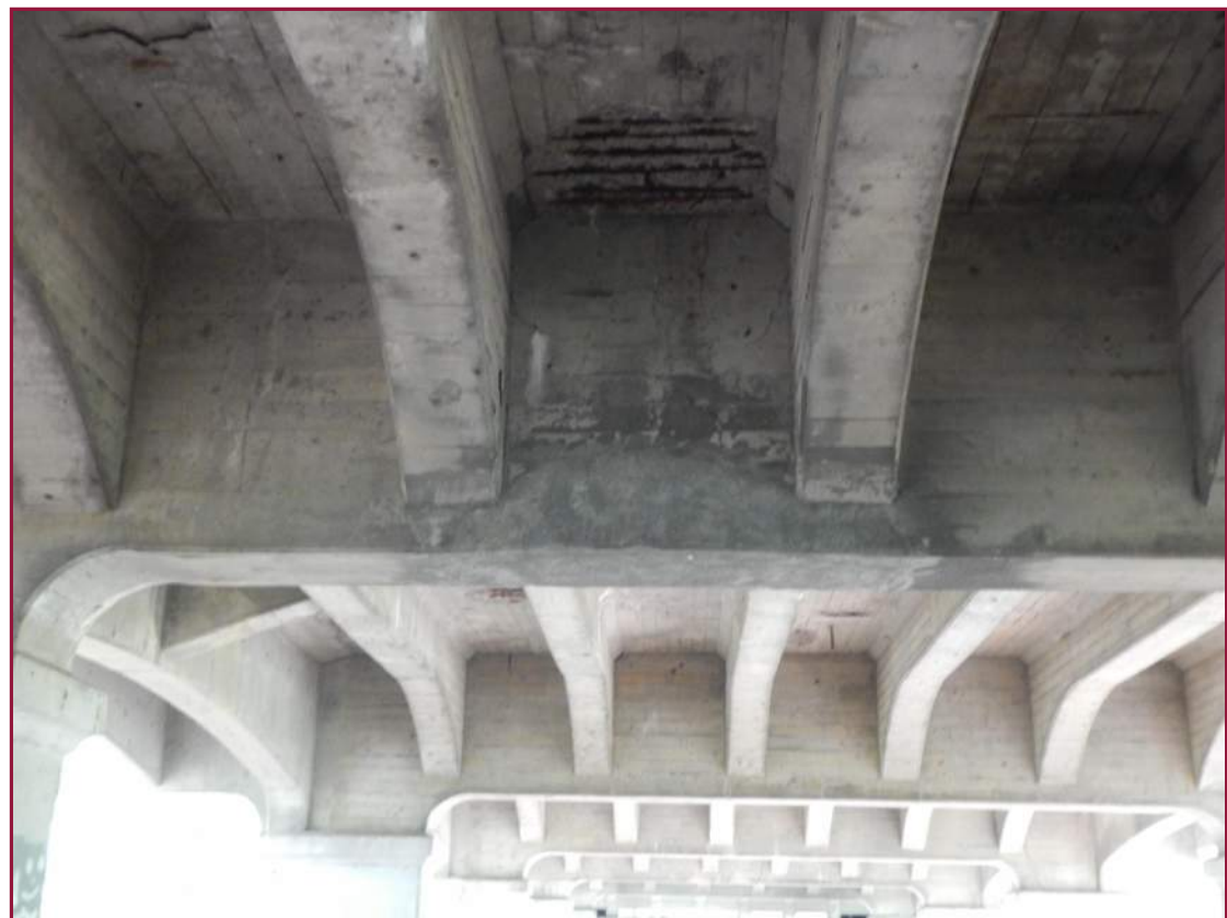
Patch in the Pier 1 cap (looking east).
