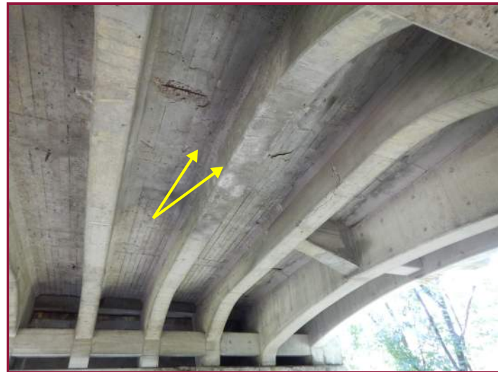
Patch to the deck underside and all faces of Beam 7 near midspan (looking southeast).
