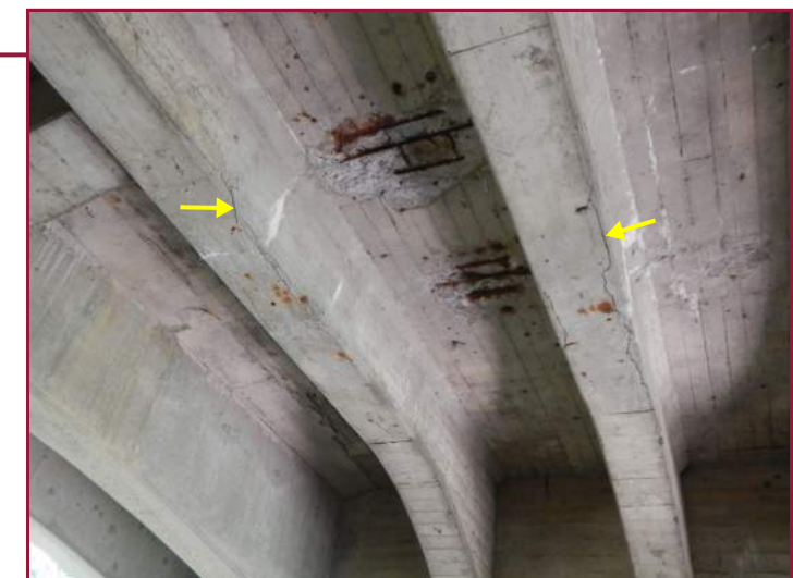
Longitudinal cracks up to 1/4" wide at delaminations in the underside of Beams 3 and 4 (looking east). Note the spalls with exposed reinforcement in the underside of the deck.
