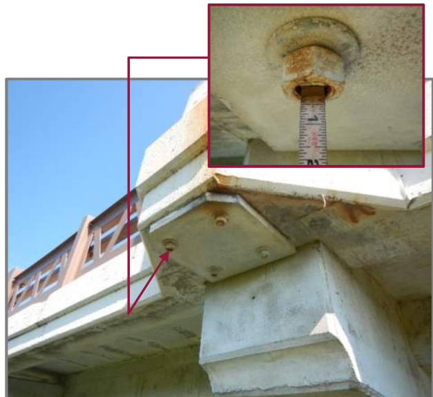
Photo 42 – Light post anchor bolts and nuts with minor corrosion and negative thread count (looking northwest at the right forward end of Span C).
