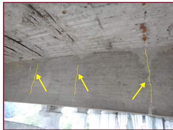
Full height vertical hairline cracks in the web on the east face of Floorbeam H5 near the midpoint (looking west).
