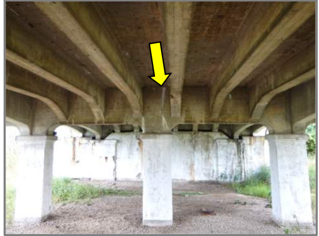
Photo 35 – West elevation of the Pier 14 cap with moderate efflorescence at full height vertical hairline cracks between Beams 5 and 6 (looking east). Note the spalls and rust staining in the Forward Abutment.
