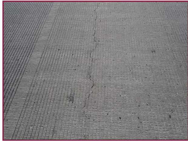
Longitudinal crack up to 1/16" wide in the eastbound lanes (looking east).
