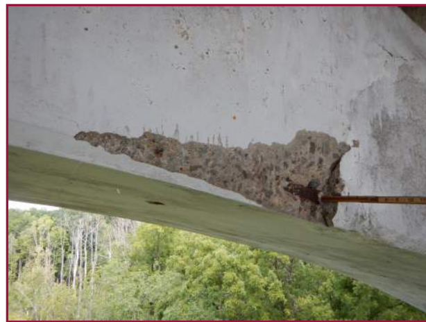
2' wide by 1' high by 2" deep spall on the south face of the North Arch below Spandrel Column 7 (looking north).
