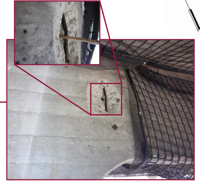
Spall with exposed and bent reinforcement in the north half of the west face of Floorbeam B9 between the Left and Right Jack Arch (looking east).
