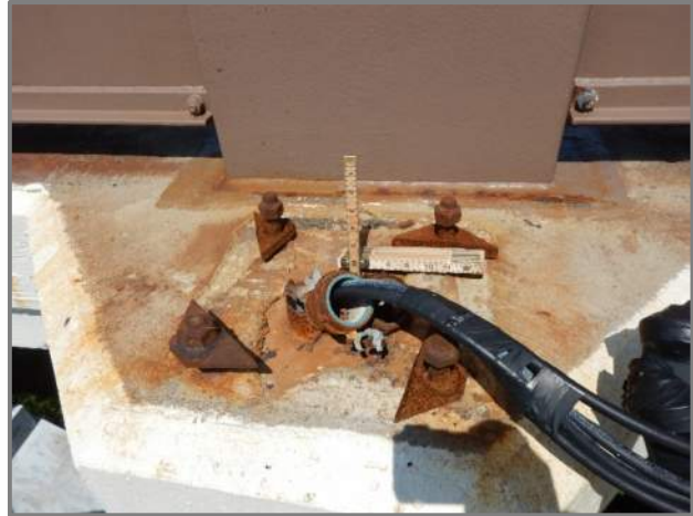
Photo 41 – Missing light post with corrosion on the anchor bolts and nuts and taped electrical wires (looking north at the right forward end of Pier 10 in Span E).
