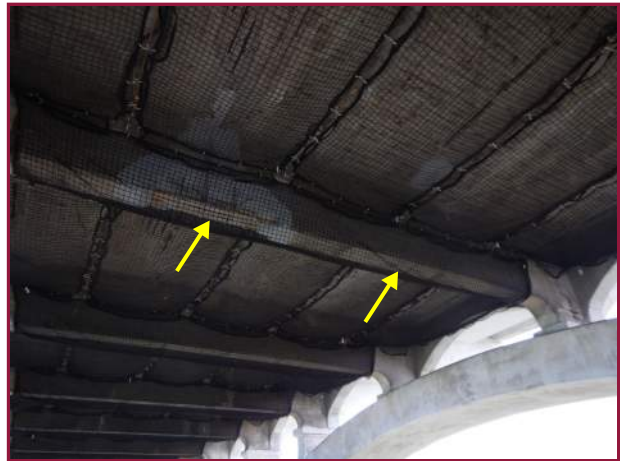
Spall with exposed reinforcement that has been sealed in the north half of the west face of Floorbeam B5 between the Left and Right Jack Arch (looking east).
