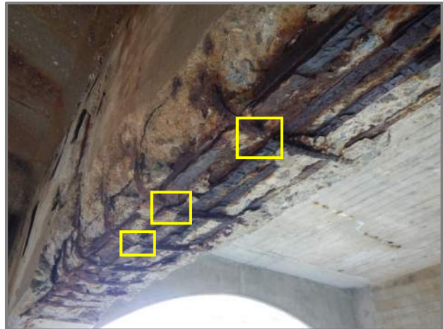
Photo 27 – Floorbeam Pier 12W spall with broken stirrups and spalling up to full height (looking southwest in Span H).
