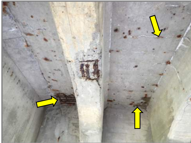
Photo 2 – Typical deck condition at the forward end of the bridge (looking east between Beams 2 to 4 at the left forward end of Span 17). Note the longitudinal construction joint between the original structure and the portion added during the major rehabilitation (typical on both sides of all spans).
