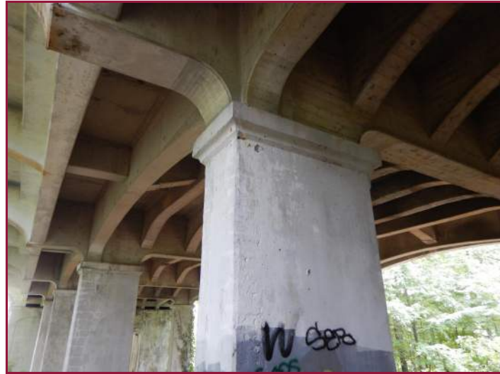
Typical hairline map cracking and minor popouts at patches in the columns (looking southeast).
