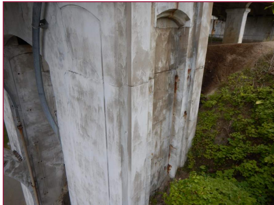
Hairline cracks with map cracking in the south face of the East Pylon right column (looking northeast).
