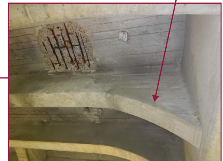
Full height vertical crack up to 1/16" wide at the east end of the Beam 4 south face (looking north).
