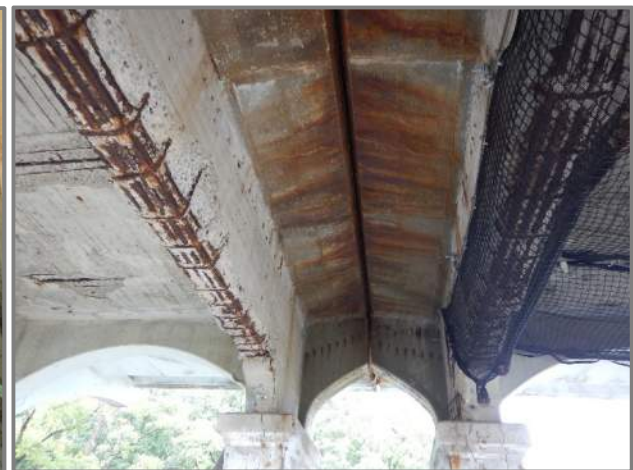
Photo 4 – Typical heavy rust staining in the deck underside below the compression joints (looking south at the Pier 6 joint underside). Note the netting in Span B and extensive floorbeam spalls.
