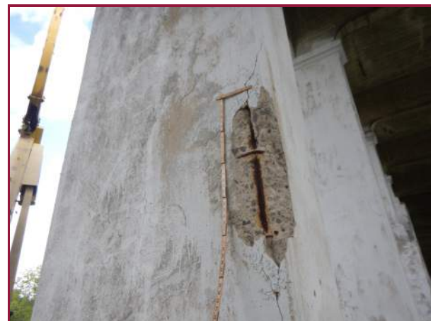
Shallow spall with exposed reinforcement on the west face of Spandrel Column 1 on the North Arch (looking east).
