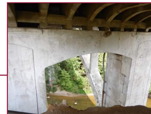
East Pylon east elevation and a spall with exposed reinforcement in the east pier cap below Beam 5 (looking west).
