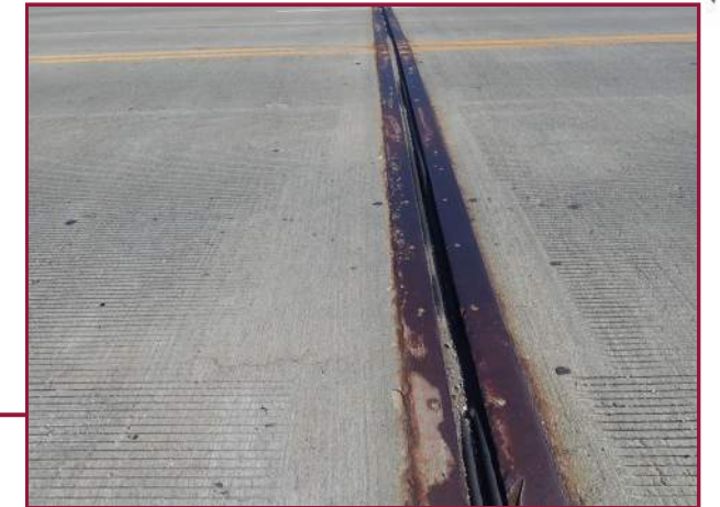
Vertical displacement of the compression seal material up to 1/4" over an 18" length (looking north).
