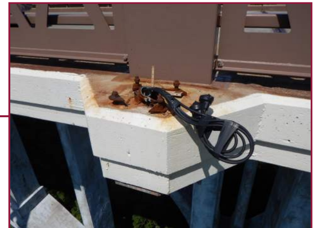
Missing light standard and wires taped off at the south railing and edge of deck at Pier 10 (looking north).
