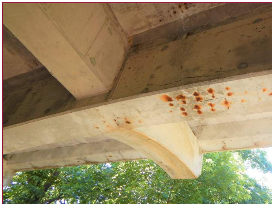
Delamination in the underside of Beam 10 near midspan (looking southeast).
