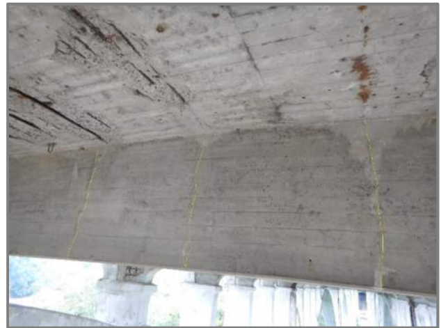
Photo 28 – Full height vertical hairline cracks in Floorbeam H5 (looking west). Cracks outlined in yellow.
