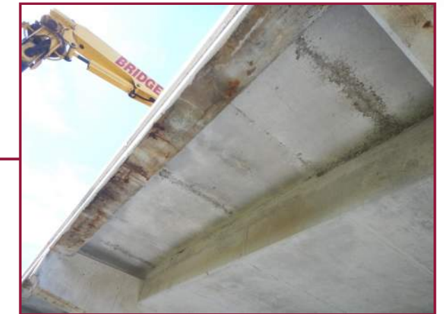
Longitudinal hairline cracks along the underside of the Right Edge Beam between Floorbeams F8 & F9 (looking north).
