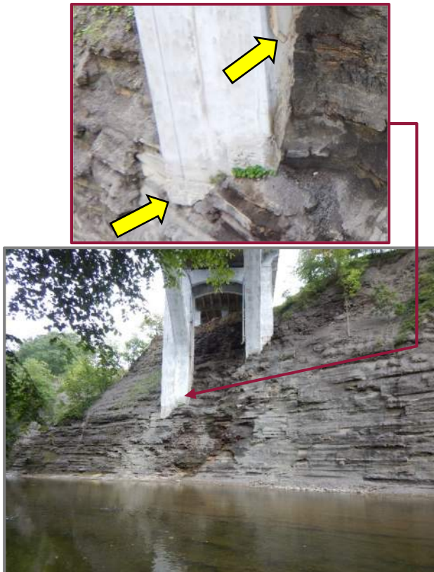
Photo 31 – Drastic elevation change between Pier 15 and the East Pylon with advanced erosion of the shale surrounding the East Pylon columns (looking east from Pier 12). Inset: Looking northeast at the left column undermined left rear corner and nearby downspout.
