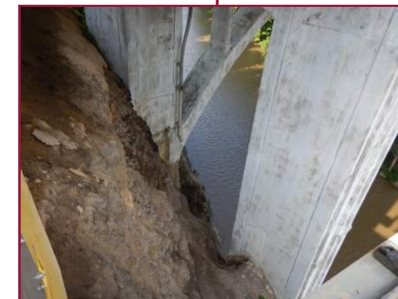
Rapid elevation change of shale slope between Pier 15 and the East Pylon (looking southwest).
