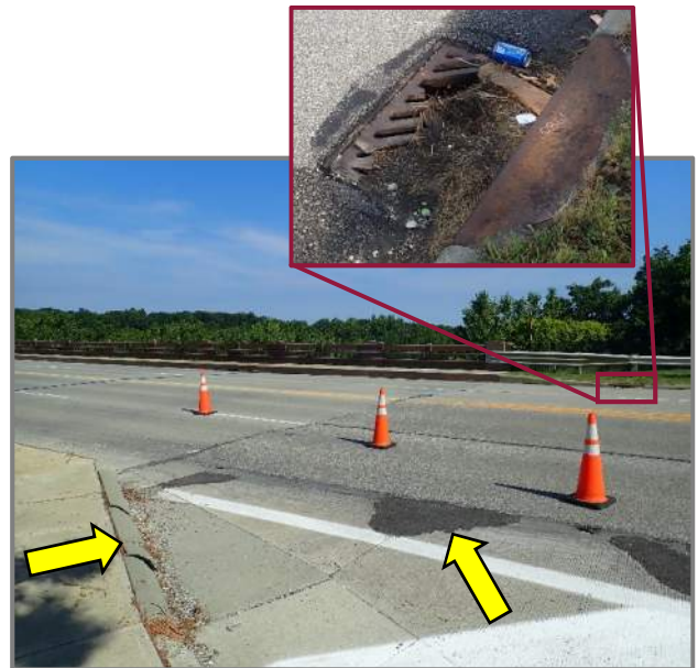
Photo 40 – Typical forward approach (looking north). Note the asphalt patches in the approach wearing surface and spalls in the right curb. Inset: Looking southwest at the cracked left forward curb inlet grate.
