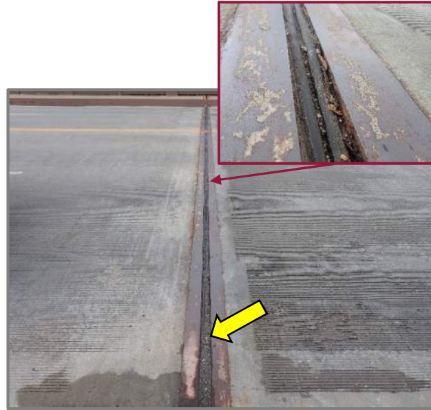
Photo 17 – Typical compression joint seal with moderate to heavy debris in the joint and laminate corrosion on the armor (looking south at the East Pylon joint). Note the heavy debris near the left curb.
