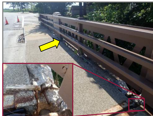
Photo 33 – Spall up to 20" deep at the rear end of the Forward Abutment right wall (looking east). Note the spalls throughout the top of the wall.
