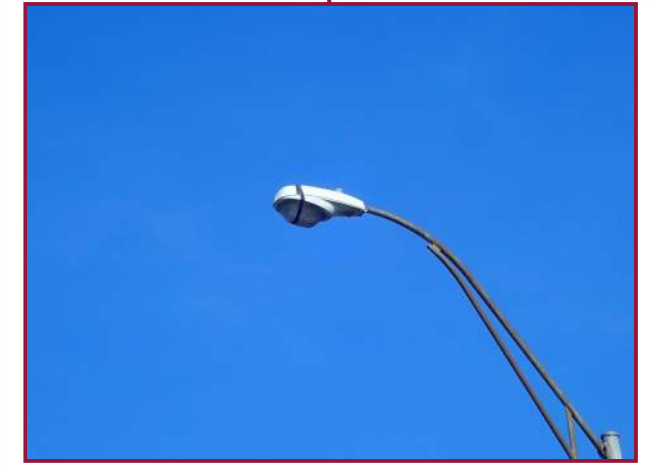
Light cover secured in closed position with tape (looking northwest). Note that the cover is hinged and is not in danger of falling.
