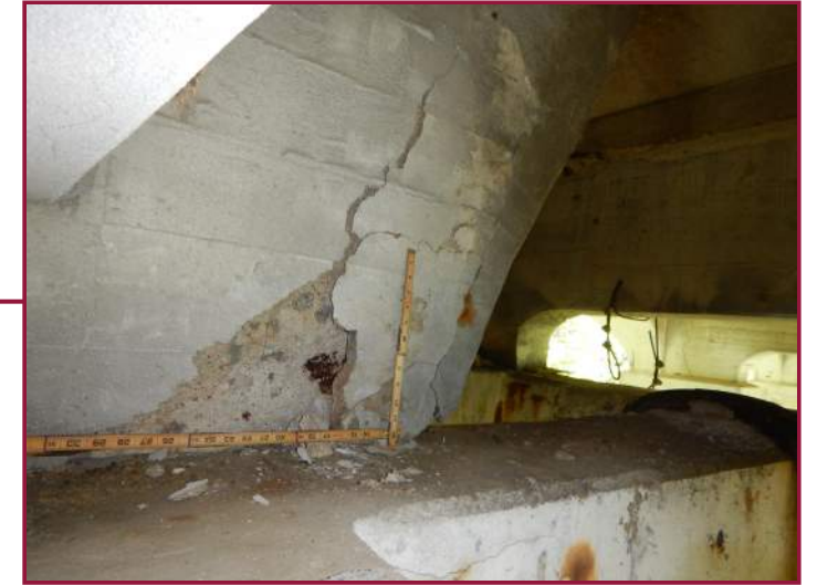
Up to 2' high by 2' long by 3" deep spall/ delamination on the south face of Beam 4 at the east end at the West Pylon (looking northeast).
