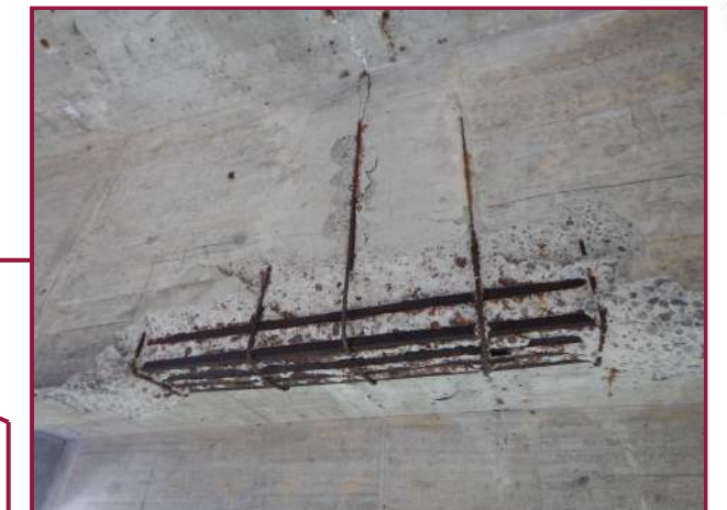
7' long by 18" high spall with exposed reinforcement and 3 broken stirrups on the east face of Floorbeam G8 at the midpoint between the Left and Right Jack Arches (looking west).
