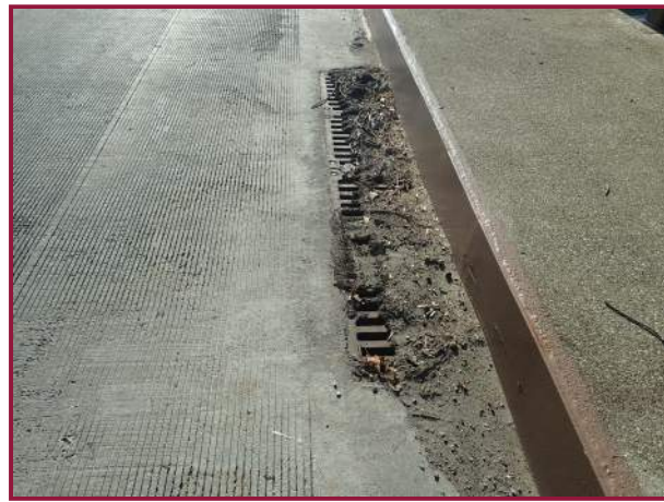
Scupper 75% blocked by debris (looking east near the right curb).
