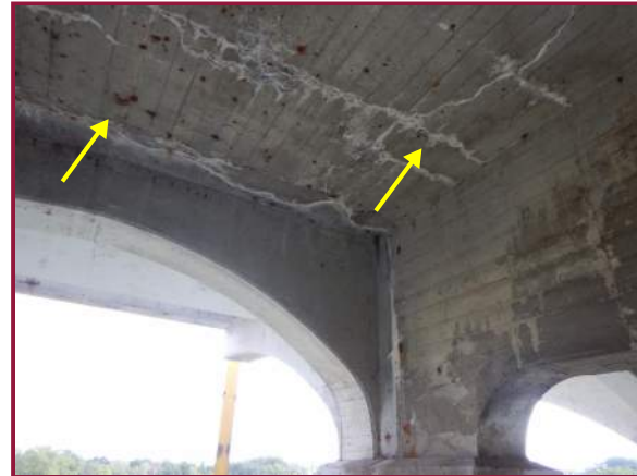
Longitudinal and transverse cracks with minor efflorescence and rust staining throughout the underside of the deck near the Left Jack Arch and west side of Floorbeam D9 (looking east).
