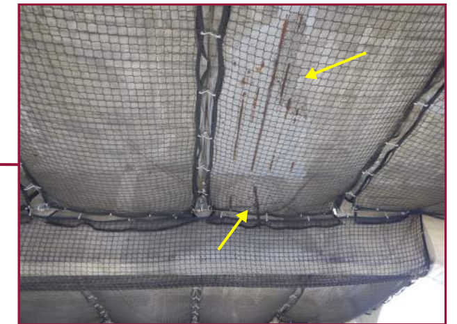
Partially sealed spalls with exposed reinforcement on the east face of Floorbeam C7 and in the underside of the deck at Floorbeam C7 (looking northwest).
