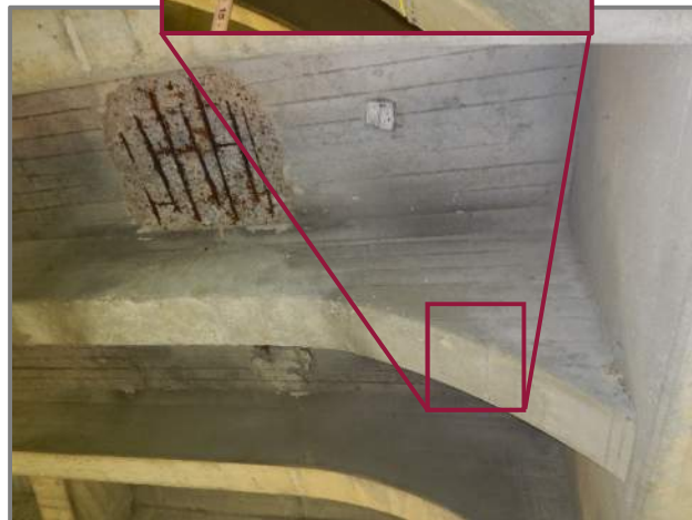
Photo 20 – 1/16" wide crack around the full perimeter of Beam 4 in Span 4 (looking north at the forward end near Pier 5). Crack outlined in yellow.
