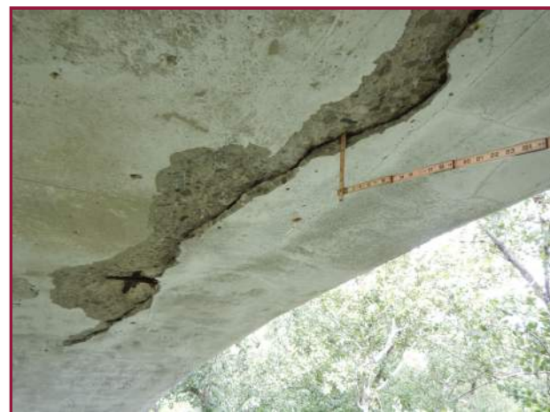
12' long by 2' wide by 2-1/2" deep spall/delamination on the underside of the North Arch between Spandrel Columns 4 & 5 (looking northwest).
