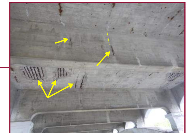
Full height vertical hairline cracks with minor spalls in the web on the east face of Floorbeam H8 near the midpoint (looking west). Note the large spalls with exposed reinforcement on the underside of the deck.
