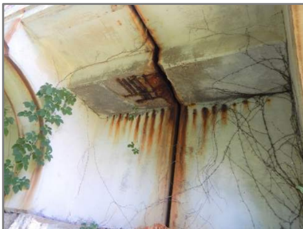
Photo 3 – Spall with three layers of exposed reinforcement at the right side of the deck underside (looking northwest at the West Pylon).
