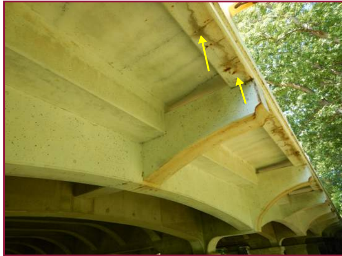
Typical longitudinal hairline cracks with rust staining and isolated spalls up to 2" deep at the north face of the Left Edge Beam near midspan (looking southwest).
