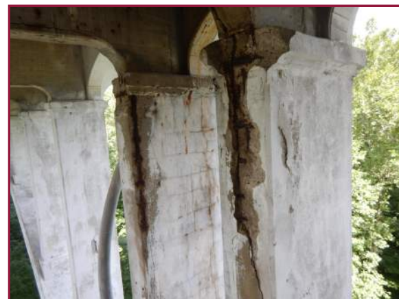
Spalls with exposed reinforcement on both columns at Pier 12 on the North Arch (looking northwest).
