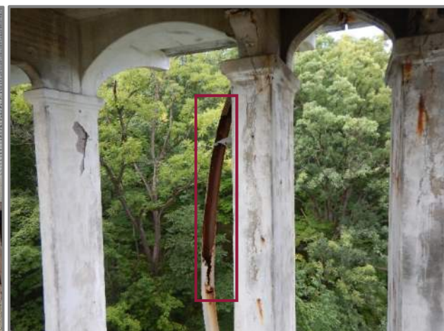
Photo 16 - 100% section loss in the downspout on the west side of Pier 6 (looking northwest).
