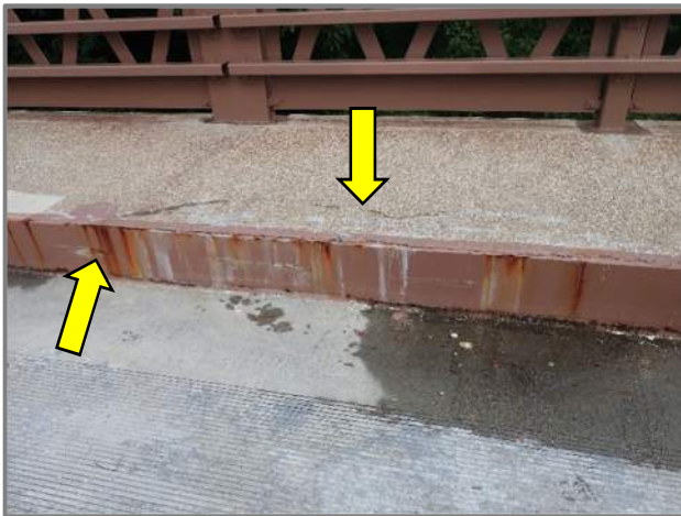
Photo 11 – Delamination at the rear end of the Span A left sidewalk (looking north). Note the typical rust staining on the curb plates at the impact scrapes and areas of failed protective coating.
