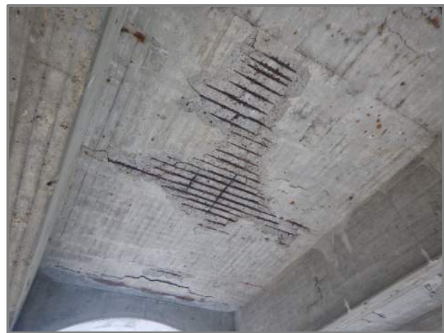
Photo 1 – Typical spalls with exposed and corroded reinforcement, delaminations, and rust staining in the deck underside (looking up and south between Floorbeams H3 and H4).
