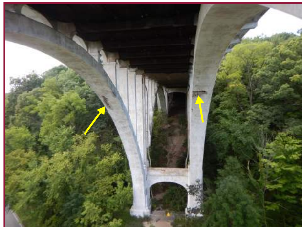
Spalls with exposed reinforcement in the underside of both the North and South Arch between Spandrel Columns 7 & 8 (looking west).
