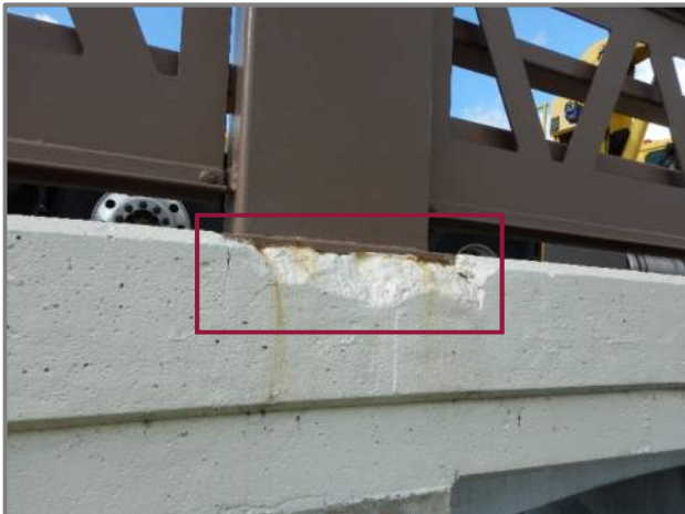
Photo 12 – Typical sealed spall in the exterior face of the concrete portion of the railings (looking southwest at the left railing near Pier 13).
