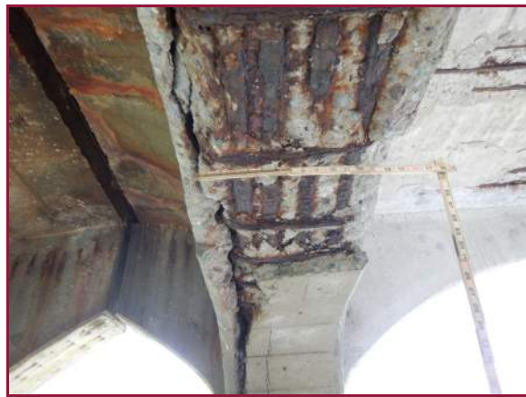
Full width spall with exposed and deteriorated reinforcement on the underside of Pier 12 near the Left Jack Arch (looking north).
