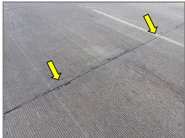
Photo 7 – Transverse cracks at the rear edge of the Rear Abutment slab wearing surface (looking southeast in the westbound lanes).
