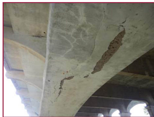
20' long by 4' wide spall/ delamination on the bottom face of the North Arch between Spandrel Columns 4 & 5 (looking east).
