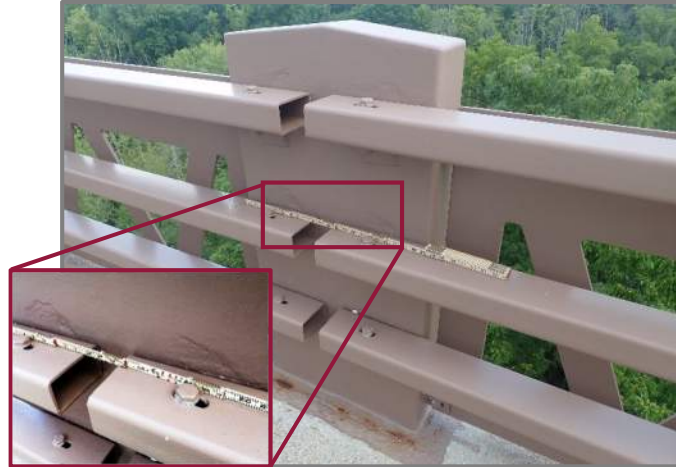
Photo 13 – Painted over pitting in a metal post above the railing (looking north at the left forward end of Span E). Note the minor corrosion at the base plate.
