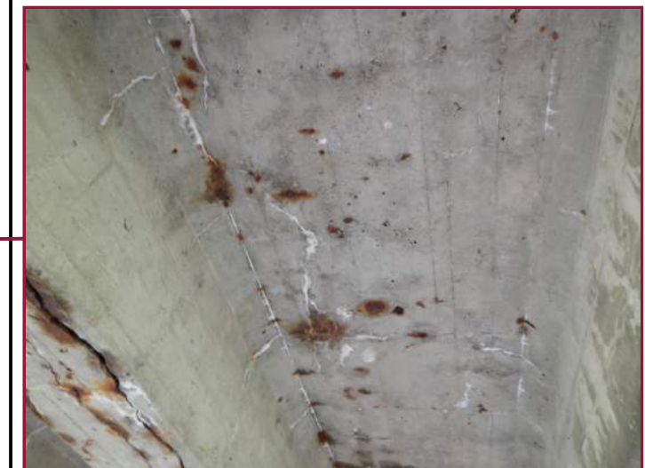
Hairline longitudinal and transverse cracks with minor efflorescence and rust staining throughout the underside of the deck between Beams 5 & 6 near the Forward Abutment (looking east).
