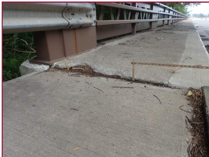
Settlement of the left rear approach sidewalk at the bridge (looking east).
