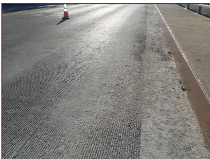
Minor scaling in the right side of the wearing surface (looking east).
