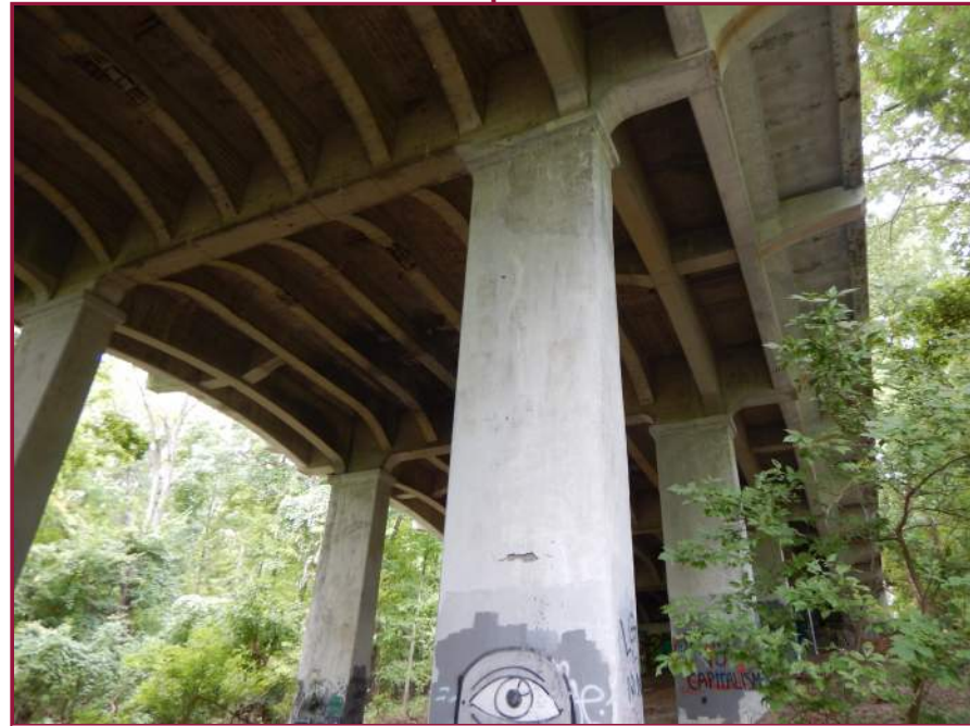
Typical hairline map cracking at patches in the approach columns (looking west).
