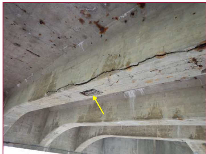
Full width delamination with an isolated spall on the underside of Beam 5 near midspan (looking north).
