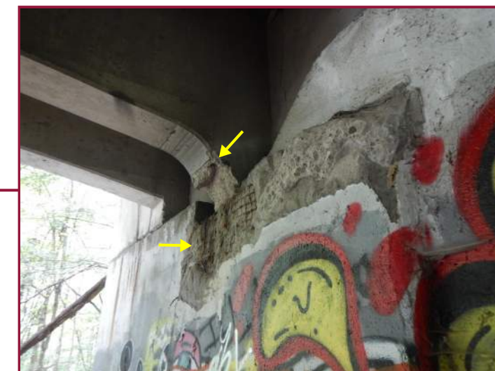
Spalls at the end of Beam 9 and in the top corner of the Rear Abutment beam seat (looking southwest).
