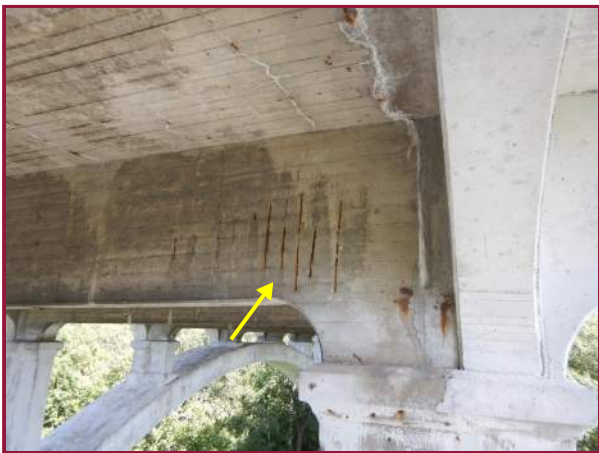
Shallow spall with exposed reinforcement due to lack of cover on the west face of Floorbeam F2 near the Right Jack Arch on the South Arch (looking east).
