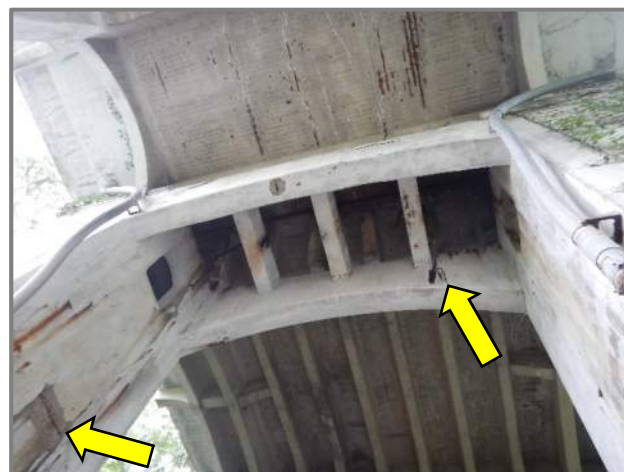
Photo 34 – East elevation of the West Pylon pier caps (looking up and west below the centerline of the bridge). Note the spall and rust staining in the West Pylon right column and the previous compression joint seal discarded on top of the pier cap struts.
