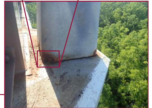
100% section loss at the bottom west corners of the light pole cover (looking east).
