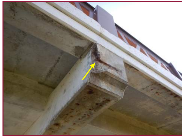
Spall with exposed reinforcement on the south face of Floorbeam C2 (looking northeast).
