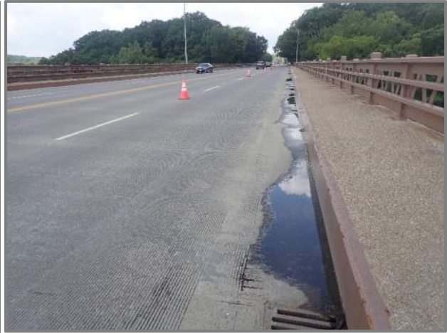
Photo 10 – Water ponding throughout the left edge of the wearing surface (looking west in the westbound lanes from Pier 7).
