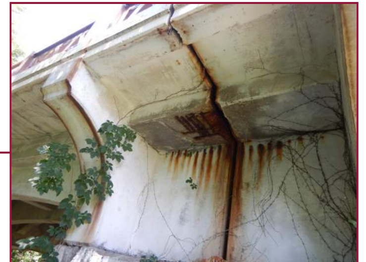
Spall with three layers of exposed reinforcement and moderate rust staining in the underside of the deck at the top of the south face of the West Pylon (looking north).
