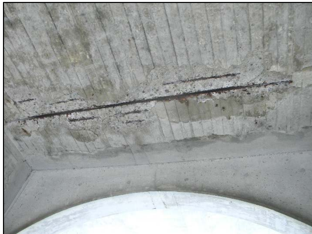
Photo 17 – Delaminations with a fresh spall near the 1989 widening construction joint. Arch F, north end of interior Bay 7
