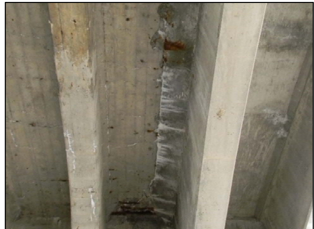
Photo 7 – Typical heavy efflorescence at construction joint. East Approach Span 9, south joint shown.
