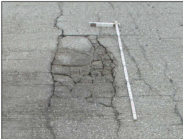
Photo 9 – Localized area of delamination that has fractured and settled 1". This location is in the East end of Arch F, center EB lane shown.
