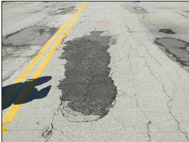
Photo 13 – The overlay is beginning to fracture and settle at the asphalt-filled spalls. Note the conchoidal breaking of the deck surface at the bottom of the asphalt patch.
