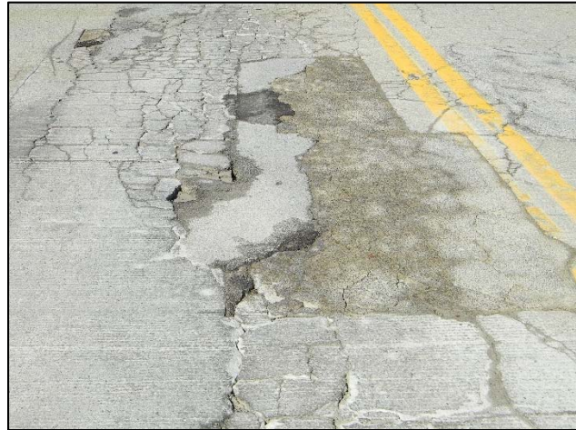
Photo 14 – Severe "block" cracking of the overlay and patches leading to fractured concrete.
