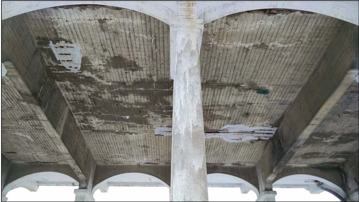
Photo 16 – Overview of Arch B, interior Bays 9 and 10, seen from the south end. Typical water infiltration and efflorescence at the cracks. Note the continuation of spalling at locations where the deck was epoxy sealed.
