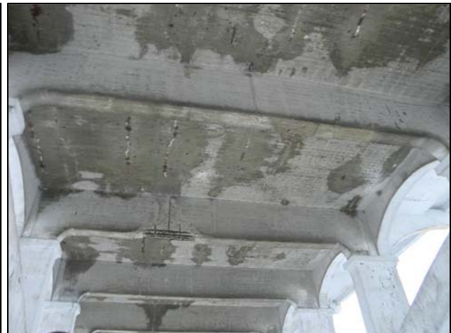
Photo 18 – General view of the bottom of Arch G deck showing extent of water infiltration.
