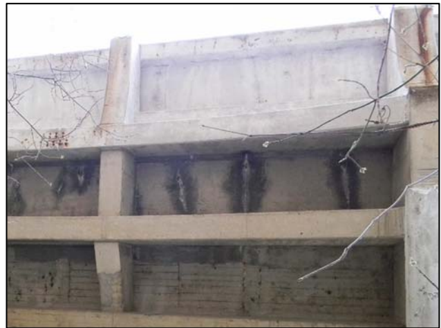
Photo 6 – Typical transverse cracks with efflorescence at 2-6 foot spacing in widened deck. Span 4, south end shown.
