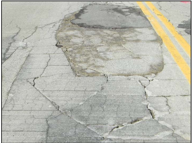
Photo 12 – Fully fractured and settled overlay and patches with a spall filled in with cracking asphalt.
