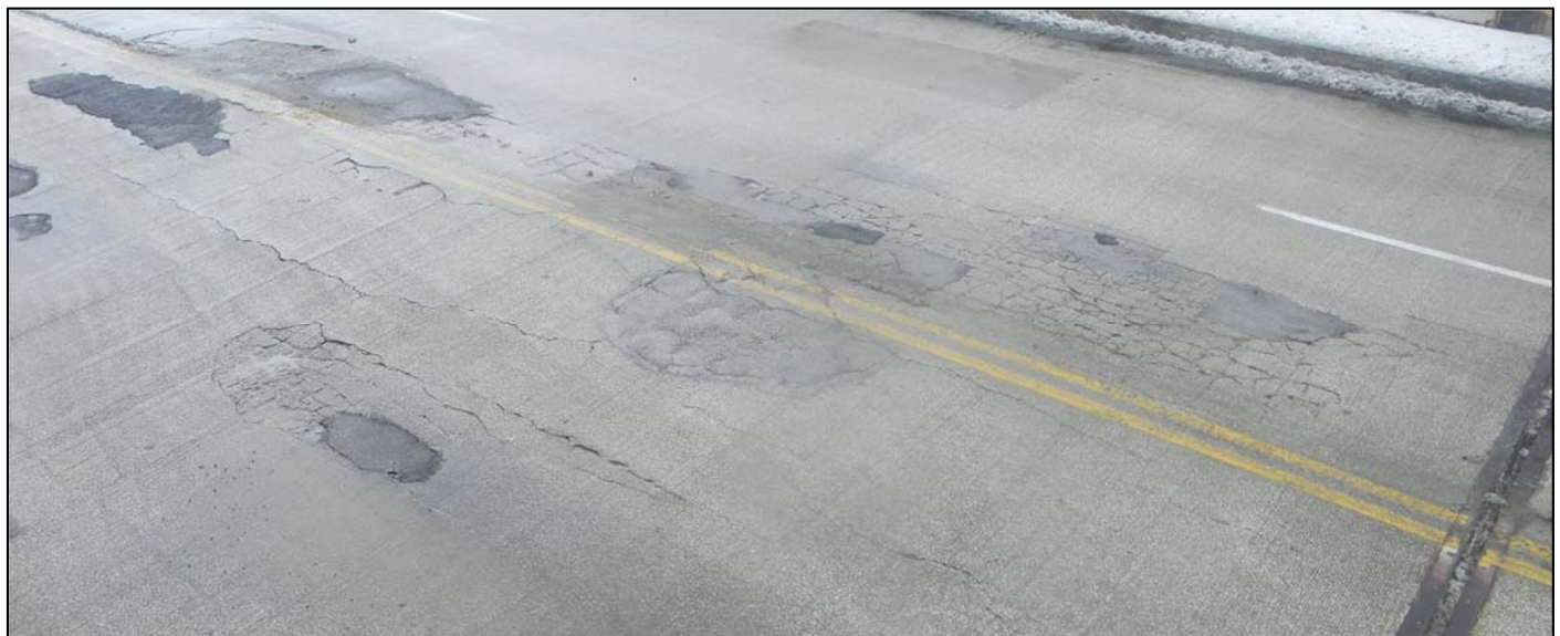
Photo 15 – Overview of the failed overlay at the west end of Arch A showing various longitudinal cracks splitting and the fracturing of the surface indicating the spalled areas are actively growing. Photo taken during the sidewalk framing inspection atop the UB-40 truck.
