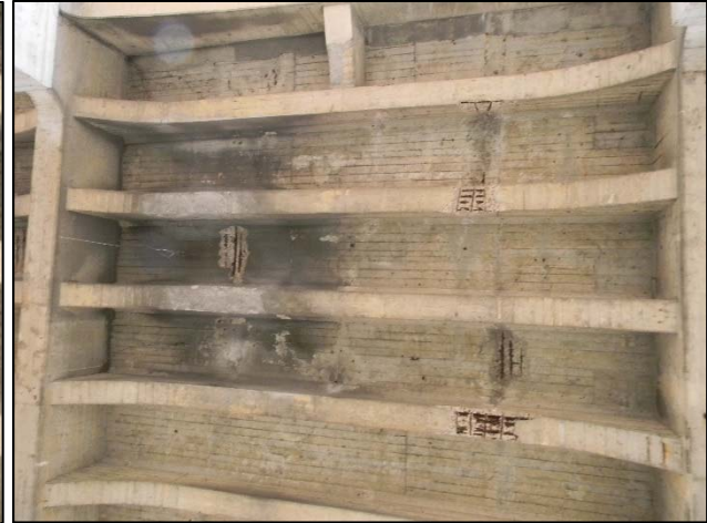
Photo 4 – Overall view of the original West Approach Span 4 underside exhibiting typical delaminations and spalling. Note extensions of spalls to the stringers.
