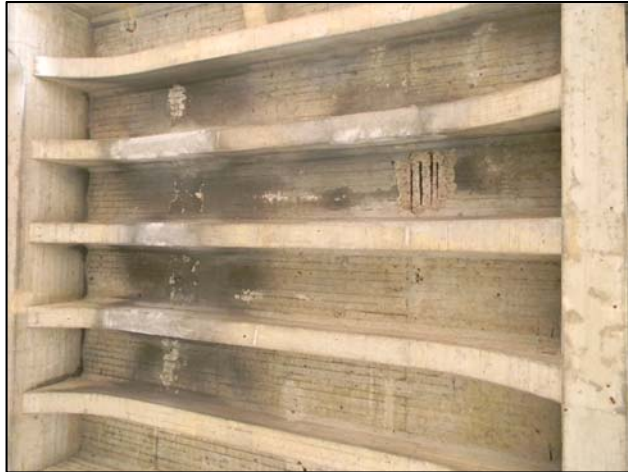
Photo 3 – Overall view of the original West Approach Span 3 underside exhibiting typical delaminations and spalling.
