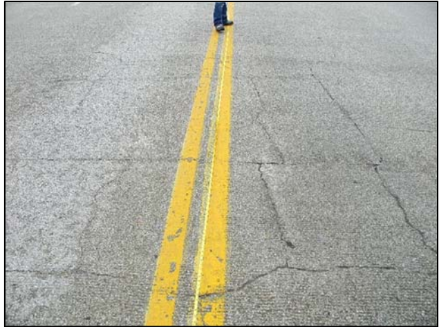
Photo 1 – Large map cracks at least 1/16" wide throughout the East Approach Spans over the original deck area.
