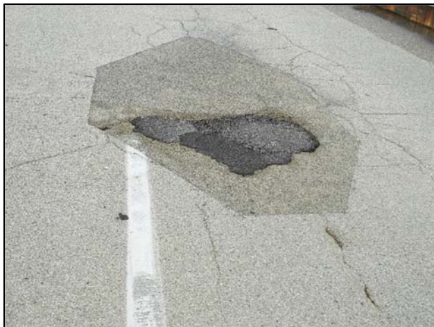
Photo 10 – Typical spall filled in with asphalt. Arch D, north EB lane shown – the surrounding area is fully delaminated and note the rust staining.
