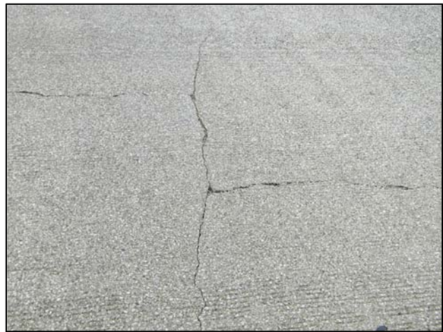
Photo 2 – Detail of irregular transverse cracks joining longitudinal cracks, typical. The overlay is typically de-bonded throughout both the East and West Approach spans in the original deck area.
