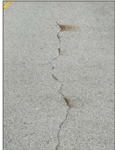
Photo 8 – Longitudinal crack exhibiting active rust staining from crack. Arch H, center WB lane shown.
