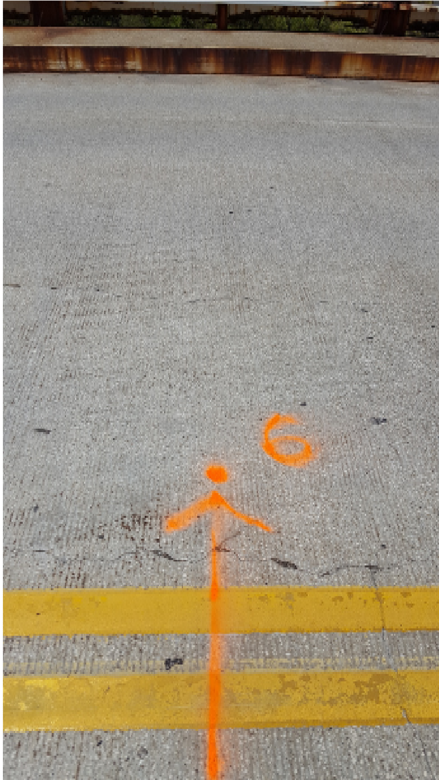
Pavement Photo C-6
