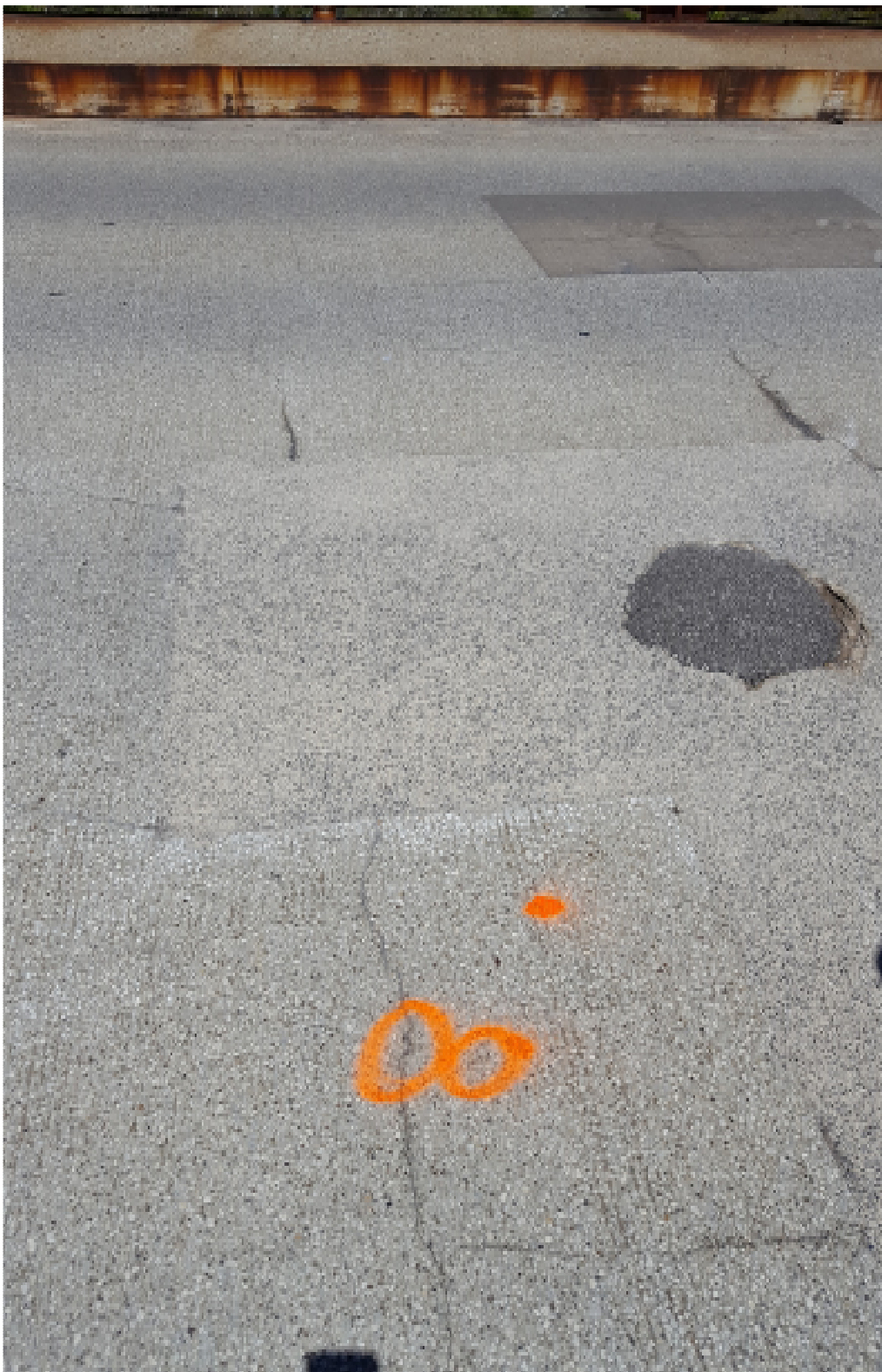
Pavement Photo C-8
