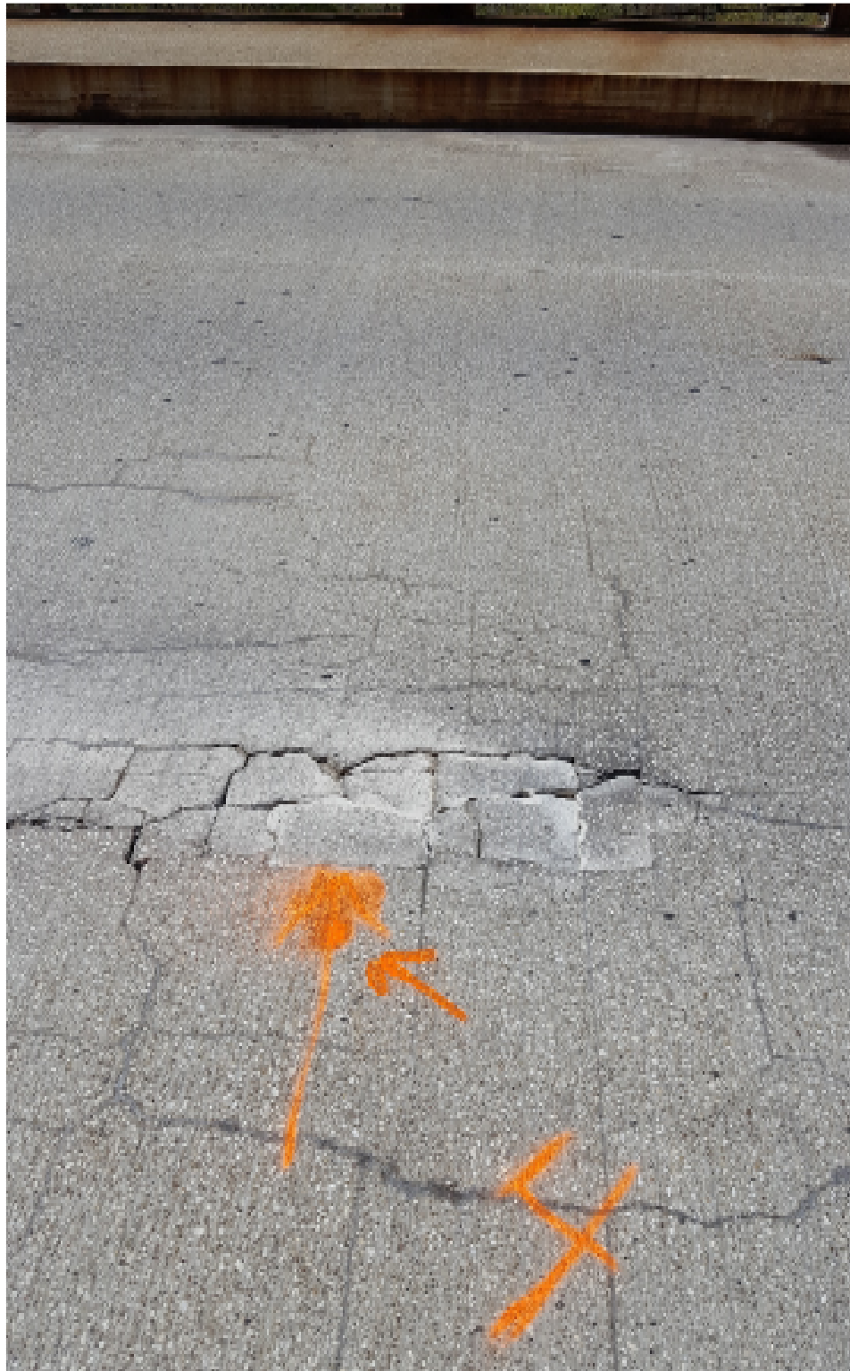
Pavement Photo C-4
