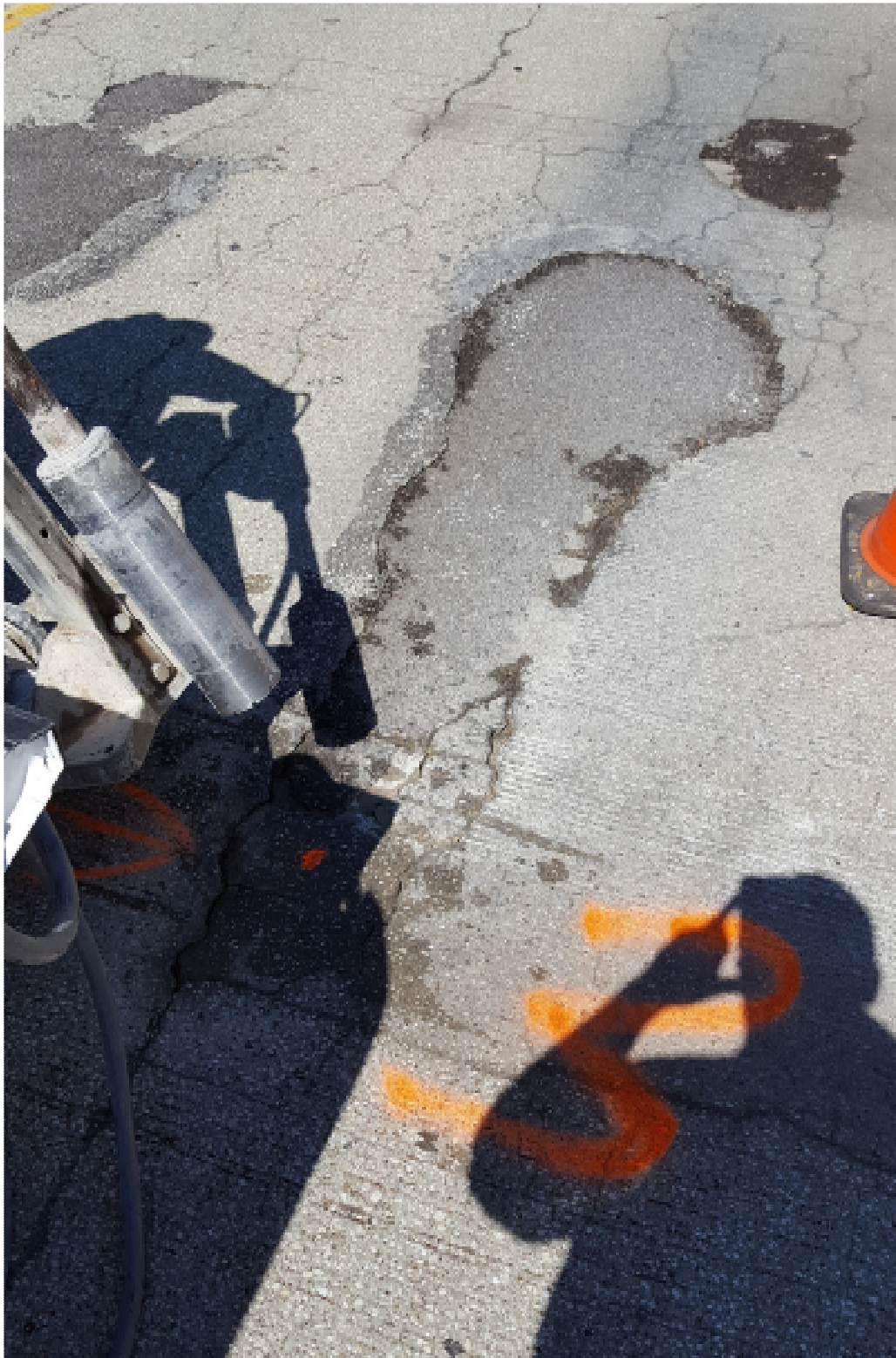
Pavement Photo C-3
