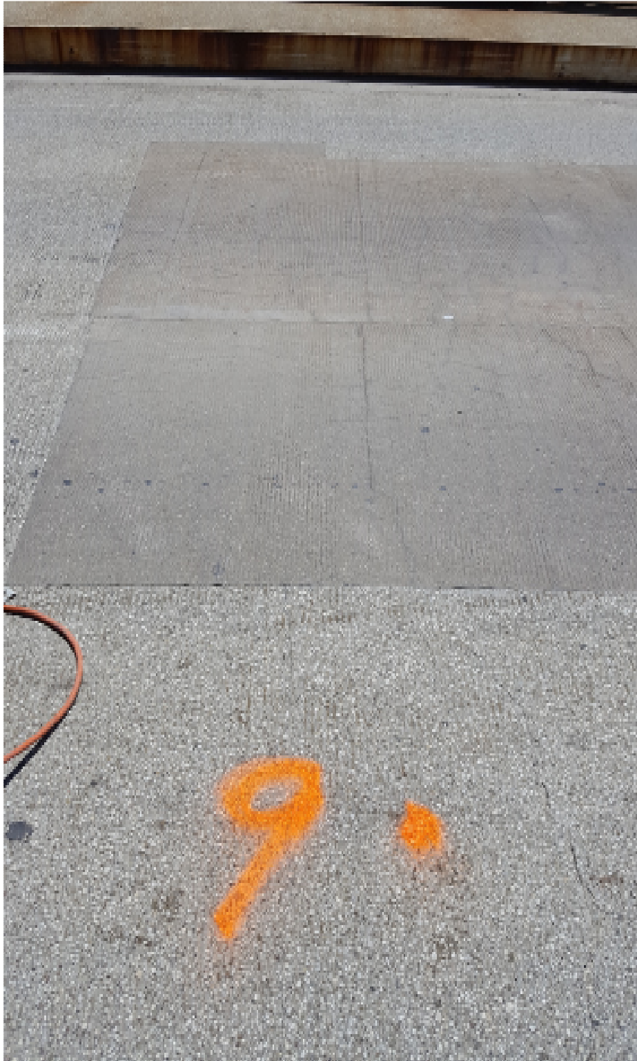
Pavement Photo C-9
