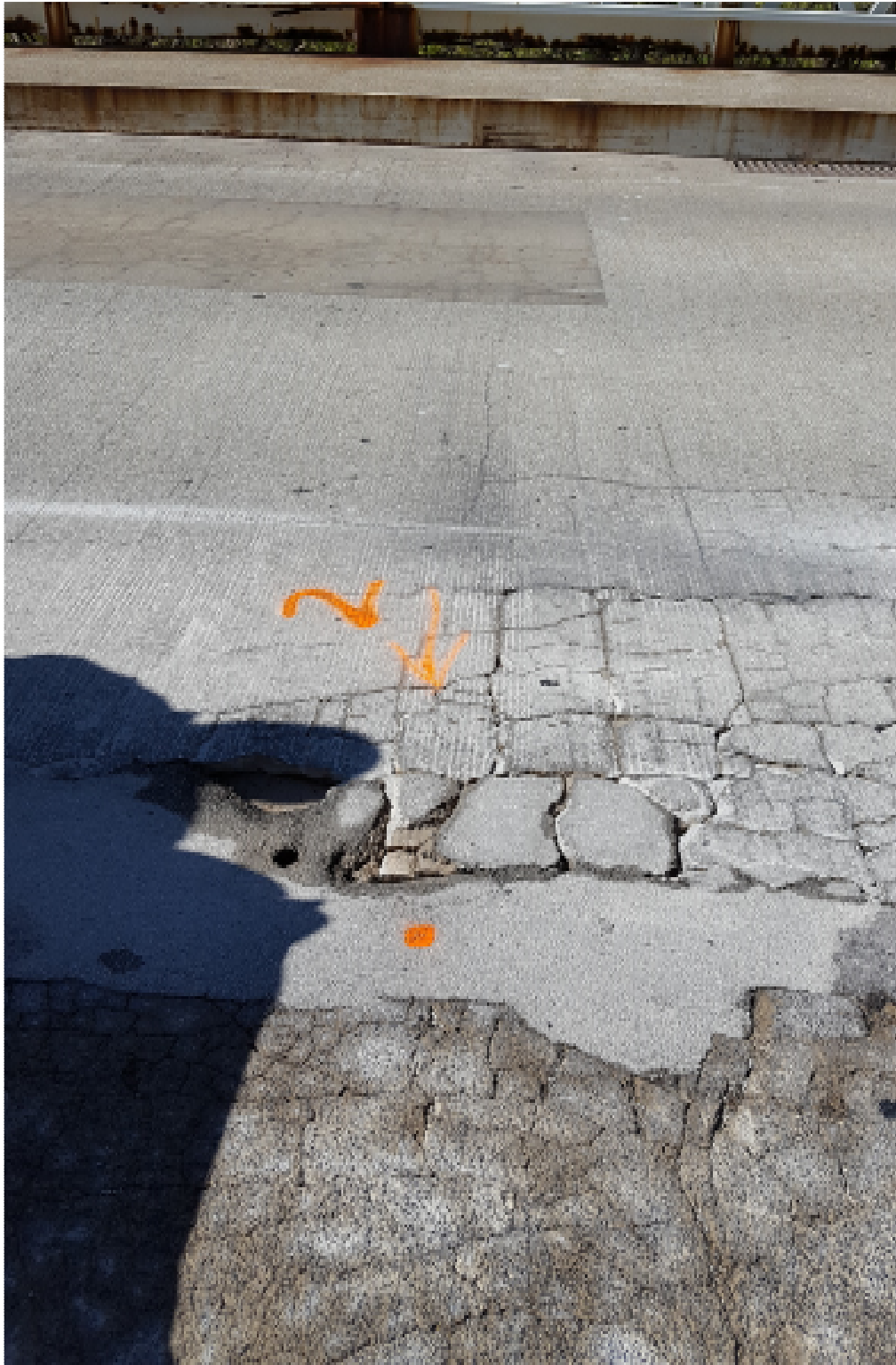
Pavement Photo C-2
