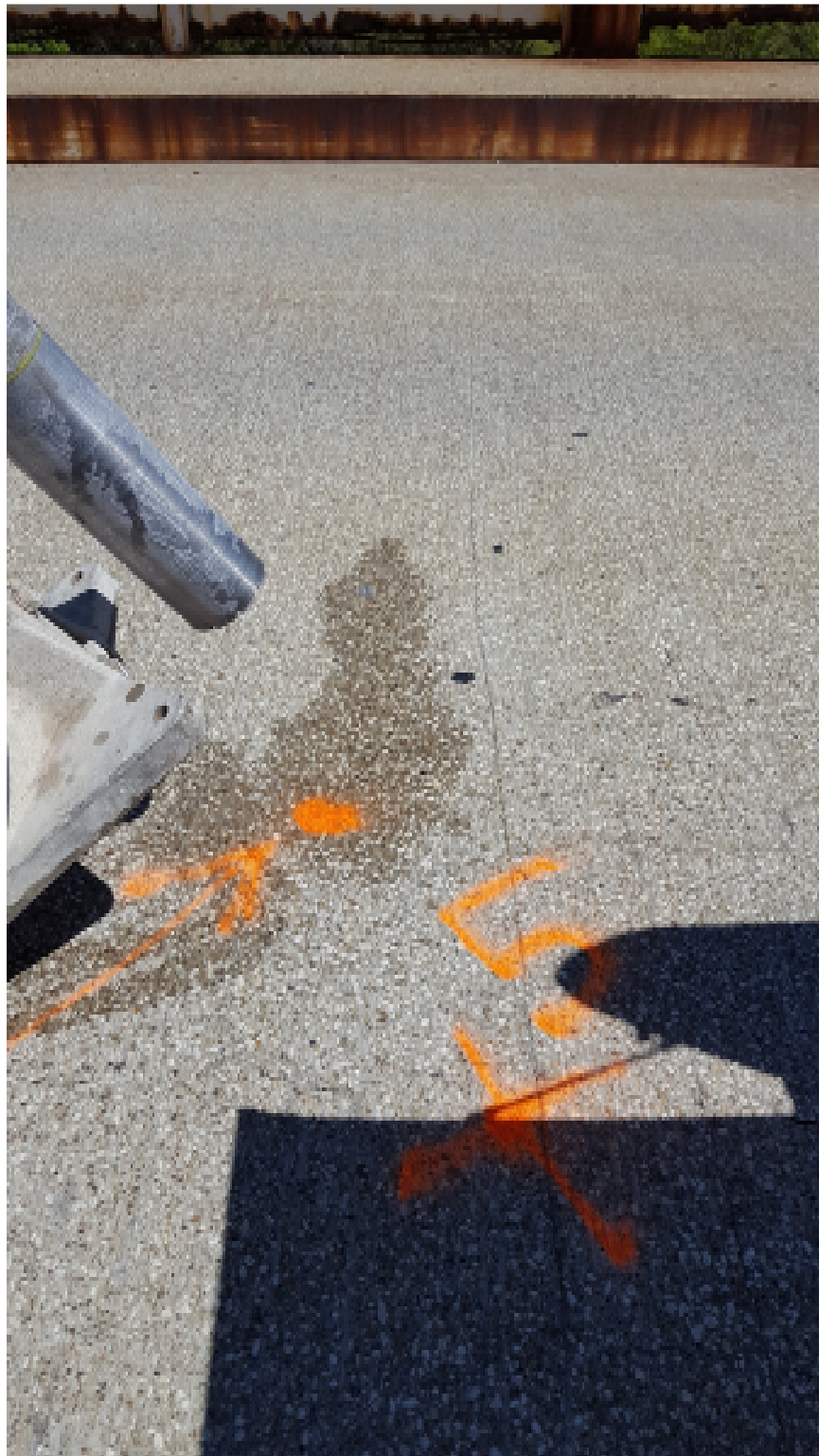
Pavement Photo C-5
