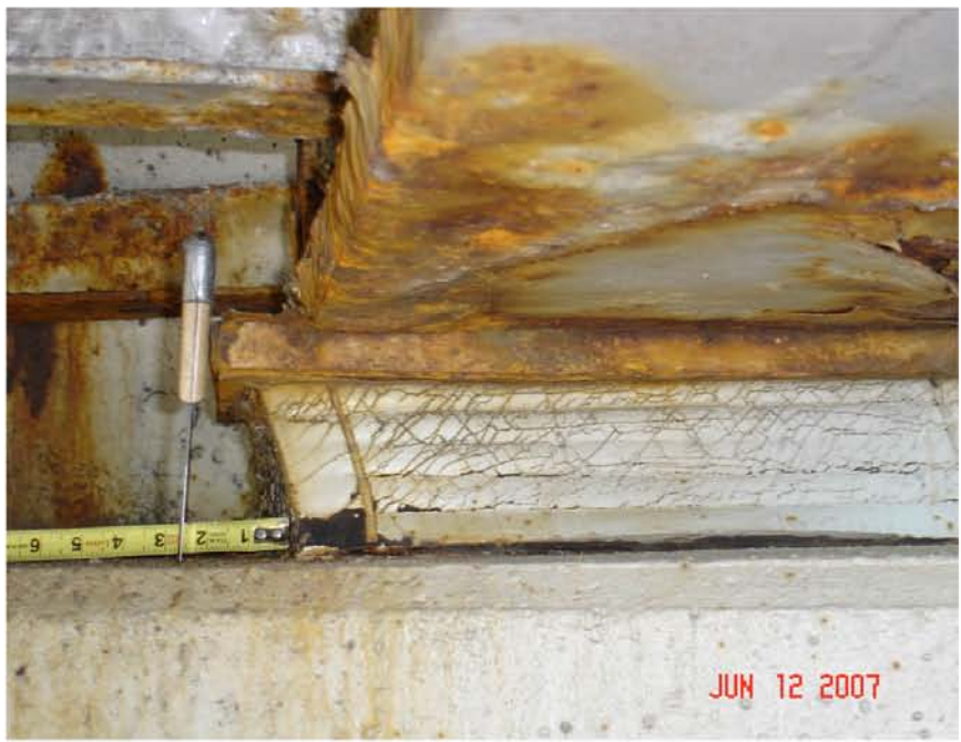
P2: NOTE THE SHIFT IN THE ELASTOMERIC BEARING. START-RIGHT BEARING.
