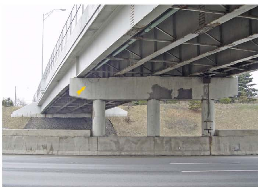
P4: ARROW POINTS TO SHEAR CRACK IN CAP OF PIER #1. LOOKING AT FINISH ABUT.
