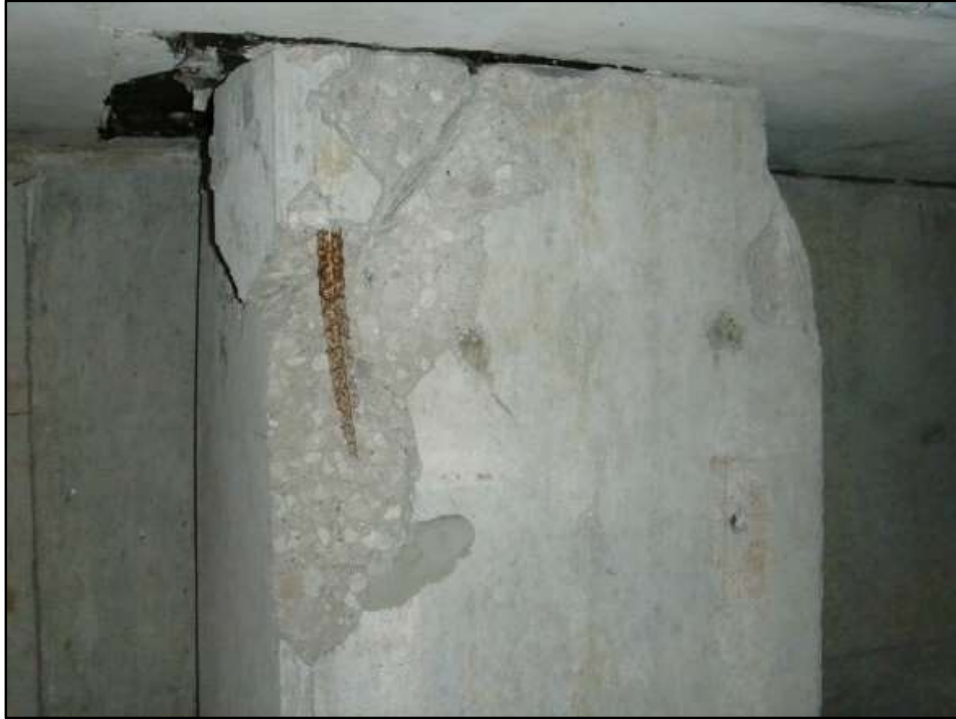
Photo 57 – Tower B Wall Shaft Wedged & Fracturing Against Sidewalk Cantilever.
