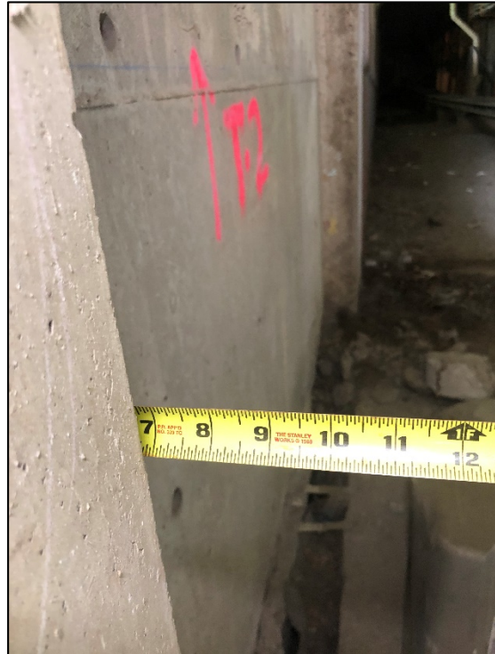
Figure 13 – GAP WAS MEASURED AT 7 INCHES JUST ABOVE THE MAIN BRIDGE LOWER DECK
