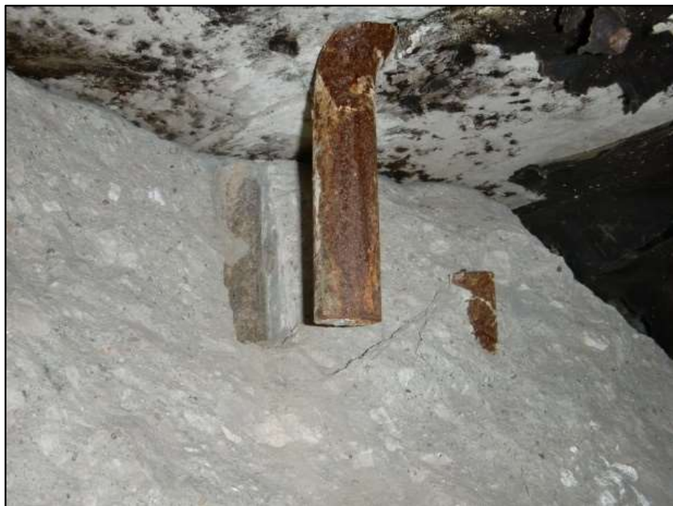
Photo 58 – Four-Inch Movement of Embedded Pipe Between Tower B Wall Shaft & Sidewalk Cantilever Above.
