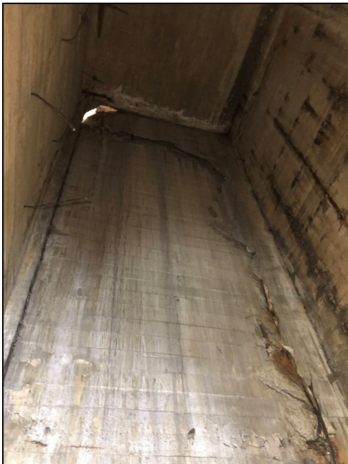
Figure 8 - EXTERIOR WALL IN EXTERIOR CELL OF MAIN BRIDGE ADJACENT TO TOWER B - SHOWING CRACKING AND PULLING AWAY OF TOWER B FROM MAIN BRIDGE. THE CEILING IN THIS PHOTO IS THE LOWER LEVEL OF THE MAIN BRIDGE
