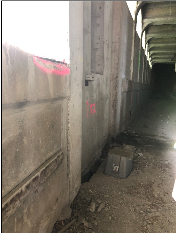
Figure 12 – TOWER B AT MAIN BRIDGE LOWER DECK LEVEL SHOWING OUTWARD MOVEMENT OF TOWER
