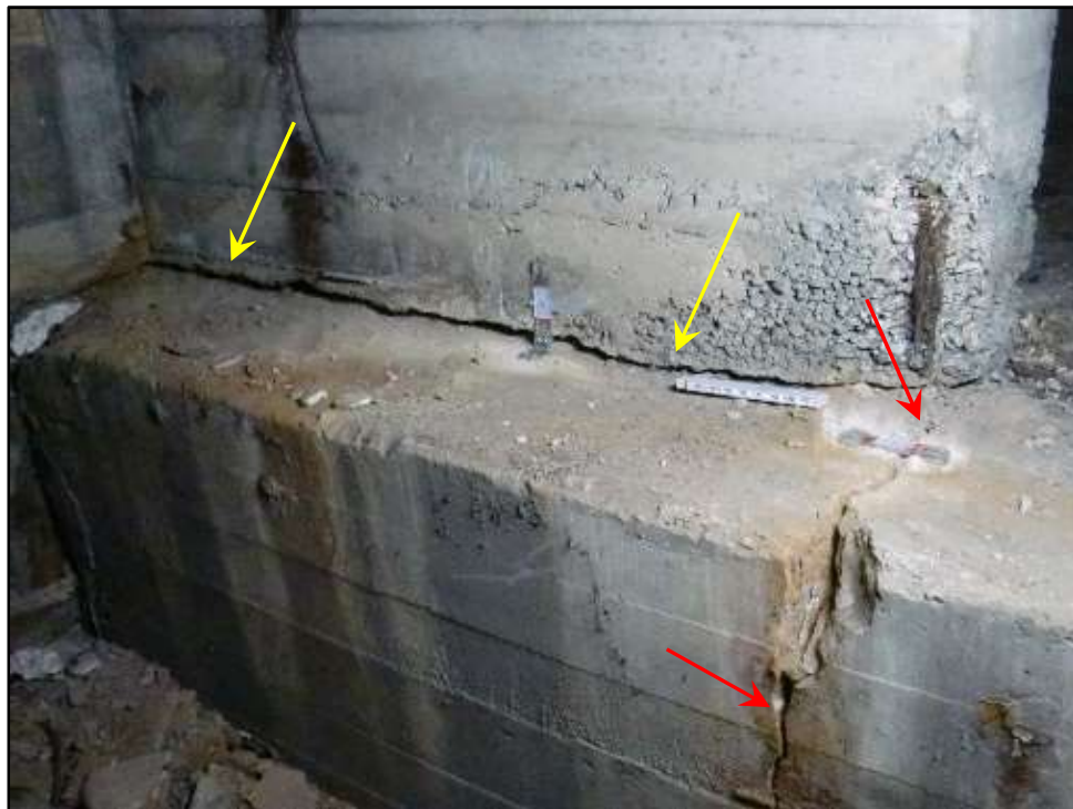
Photo 56 – Tower B Footing Crack (Highlighted with Red Arrows), and Footing Rotation & Drop with Respect to Transverse Wall (at Yellow Arrows), Looking South.
