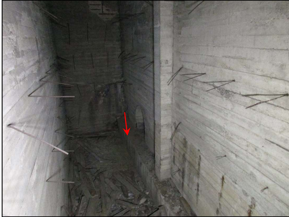
Photo 55 – Location of Tower B Footing Crack (at Arrow), Looking South in Cellular Construction, Panel 2, Span 1B.
