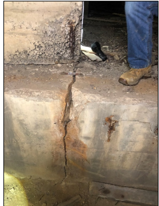
Figure 9 - FOOTING ADJACENT TO MOUSEHOLE IN EXTERIOR CELL OF MAIN BRIDGE. SHOWING CRACK. THIS IS THE POINT OF ROTATION OF TOWER B.
