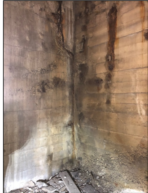
Figure 7 - INSIDE OF BRIDGE (AT BASE) – CRACKING OF EXTERIOR WALL AT LEFT WHICH IS ADJACENT TO TOWER B INSIDE WALL
