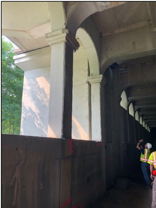
Figure 10 – TOWER B AT SEEN FROM THE LOWER DECK, ALSO SHOWING THE MAIN BRIDGE CANTILEVERED FLOOR BEAMS WHICH SUPPORT THE SIDEWALK, INDEPENDENT OF THE TOWER
