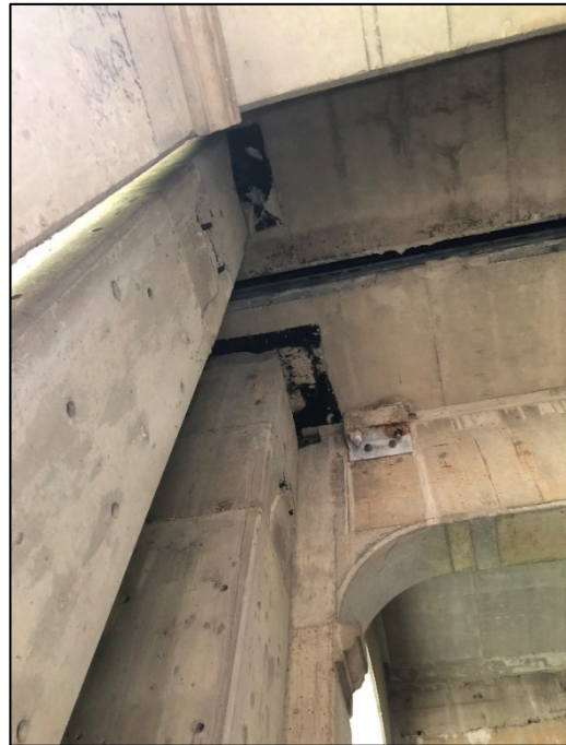
Figure 11 – TOWER B RECTANUGALAR COLUMNS ADJACENT TO MAIN BRIDGE COLUMNS. ALSO SHOWN IS THE OUTWARD DEFLECTION AT THE BOTTOM OF THE MAIN BRIDGE TOP DECK, AND THE BOND BREAKER AT THE TOP OF THE TOWER B COLUMNS.
