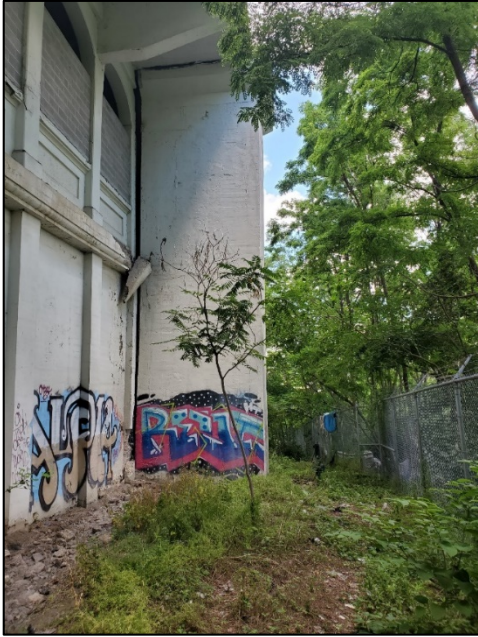
Figure 6 – TOWER B (LOOKING UPSTATION) – ROTATION OF TOWER AWAY FROM MAIN STRUCTURE
