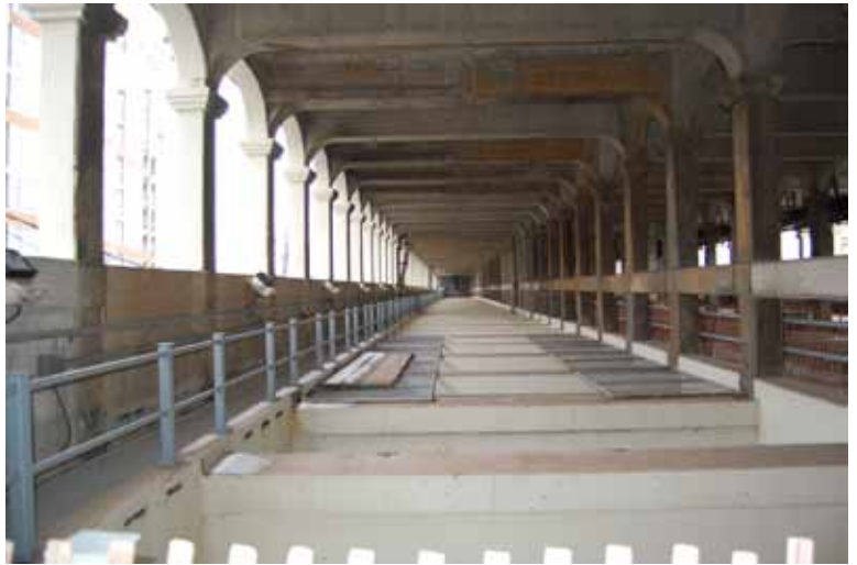
CANTILEVERED SECTIONS OF THE BRIDGE have an open decking system that would need to be fenced off or partially covered to prevent people from gaining access or falling through.
