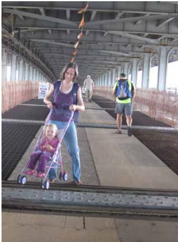
PLYWOOD SURFACE over the grated deck at the center span is difficult to navigate with bicycles, wheelchairs, and strollers. A continuous, non-skid surface needs to be installed to provide full accessibility across the bridge.
