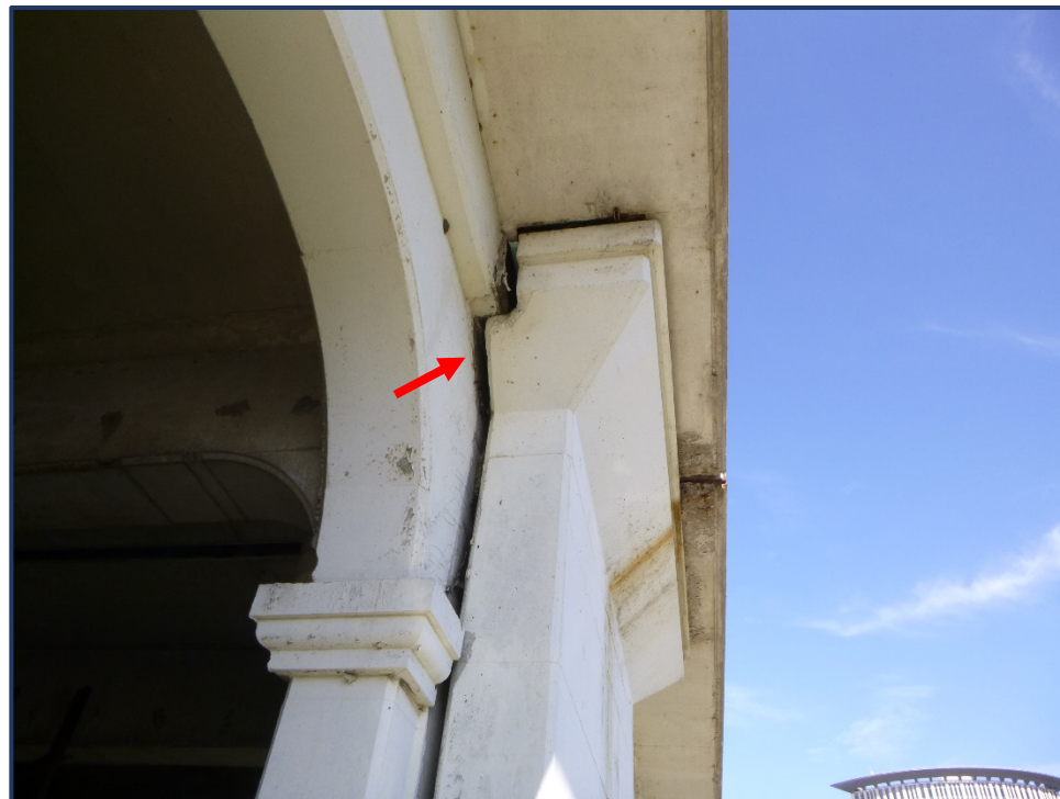
Photo 205-6 – Pier 6, South Tower Leaning Away from Bridge at Top
