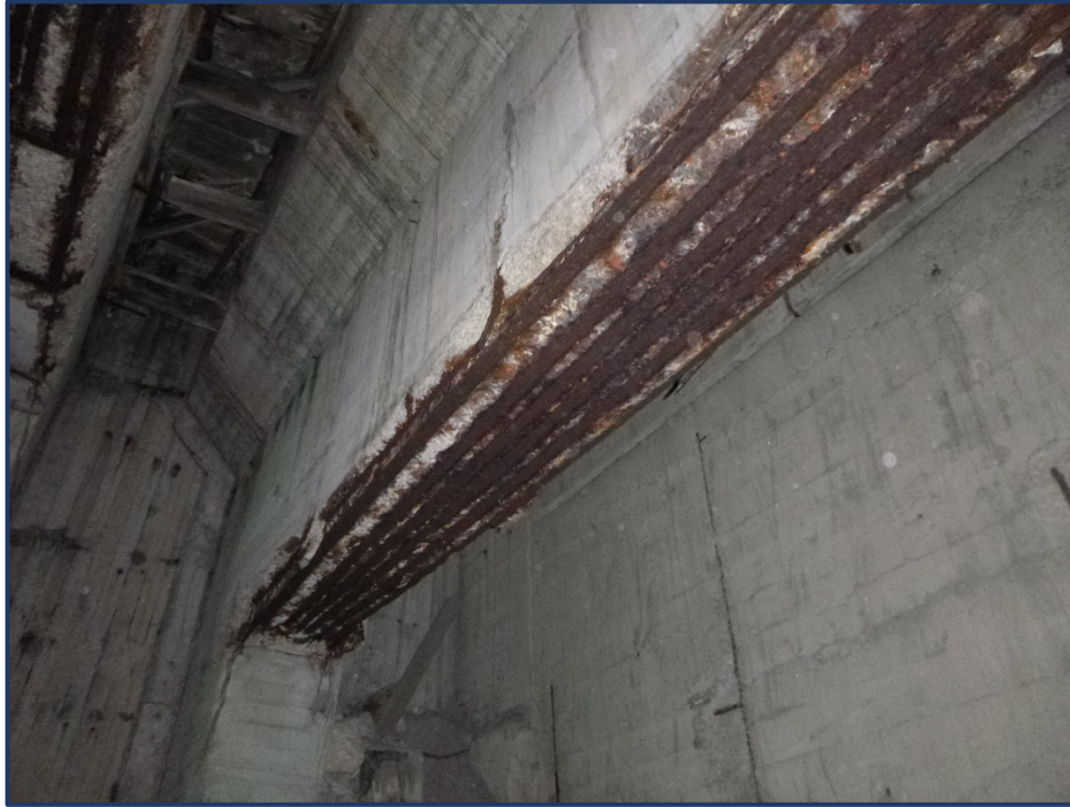
Photo 155-5 – East Abutment Chamber Floorbeams, Typical Spalling with Deteriorated Reinforcing
