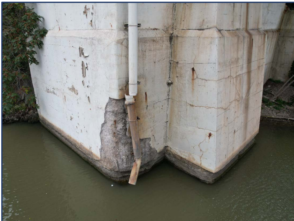
Photo 210-2 – Pier 3, Southeast Corner, Spalling and Delamination at Waterline
