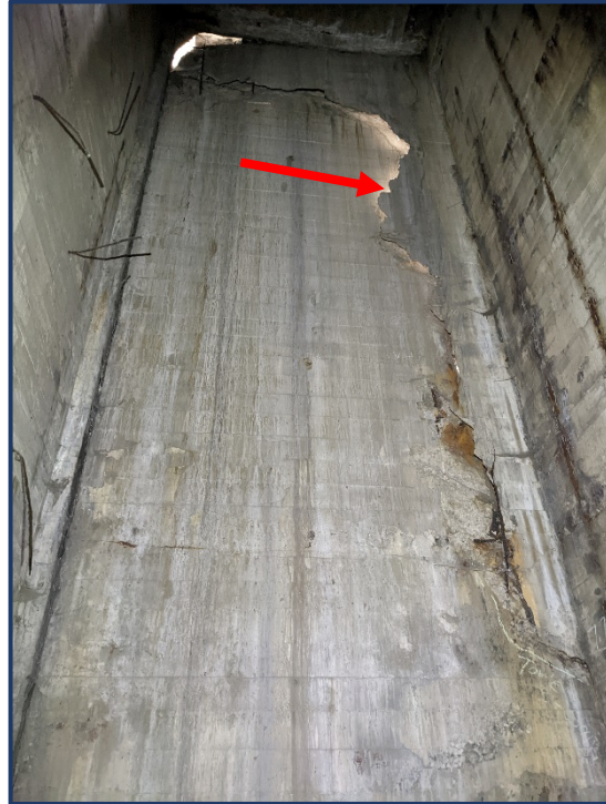
Photo WW-2 – West Abutment Chamber, Crack Through Wall at Tower B
