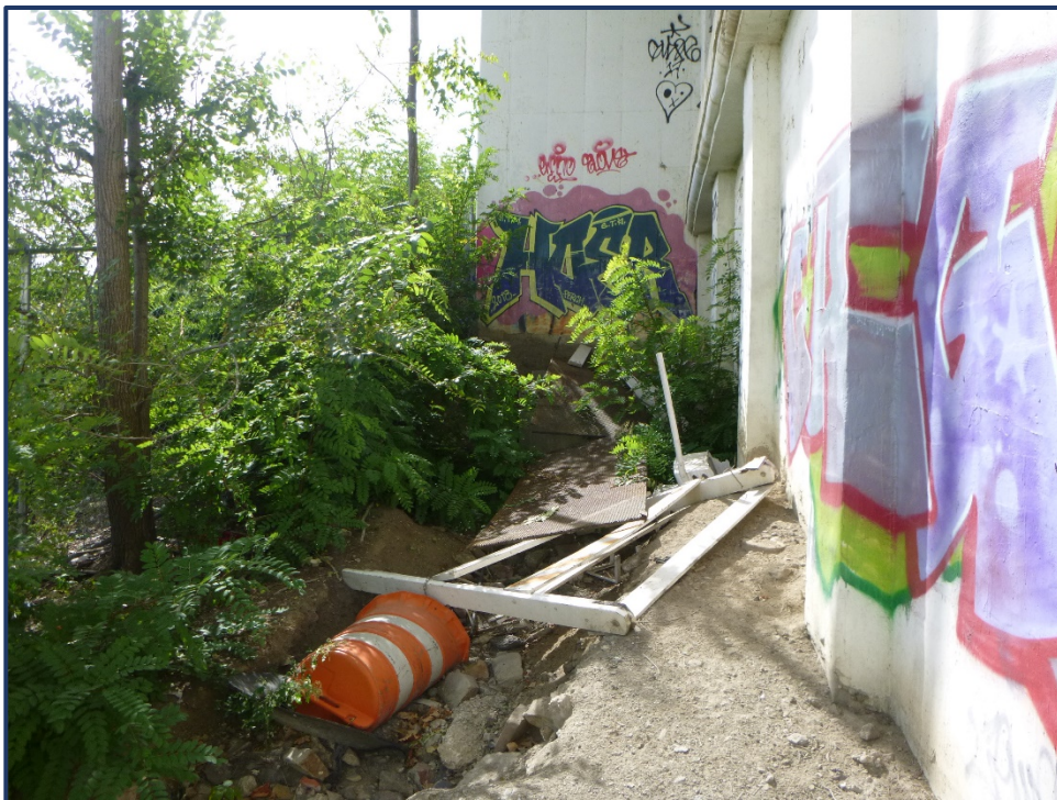
Photo APR-2 – Erosion Channel with Debris on South Side of Span 1A
