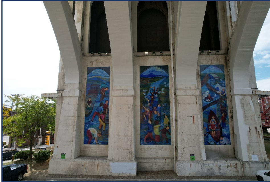
Photo 210-1 – Pier 4, East Face, Typical Map Cracking in Lower Portion
