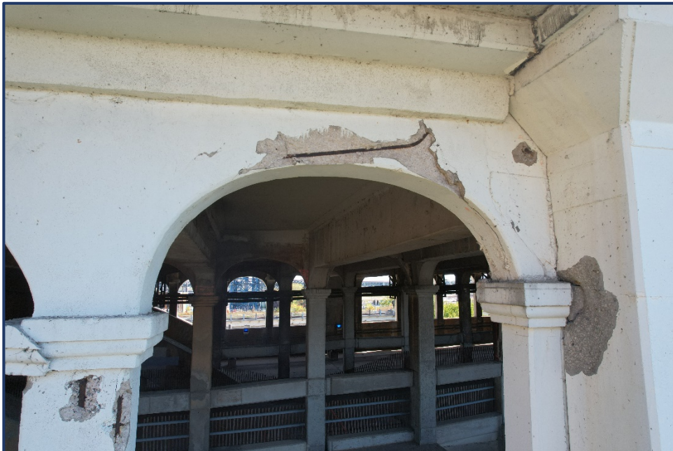
Photo 144-7 – Span 12, North Exterior Arch, Spalling with Exposed Reinforcing of Jack Arch
