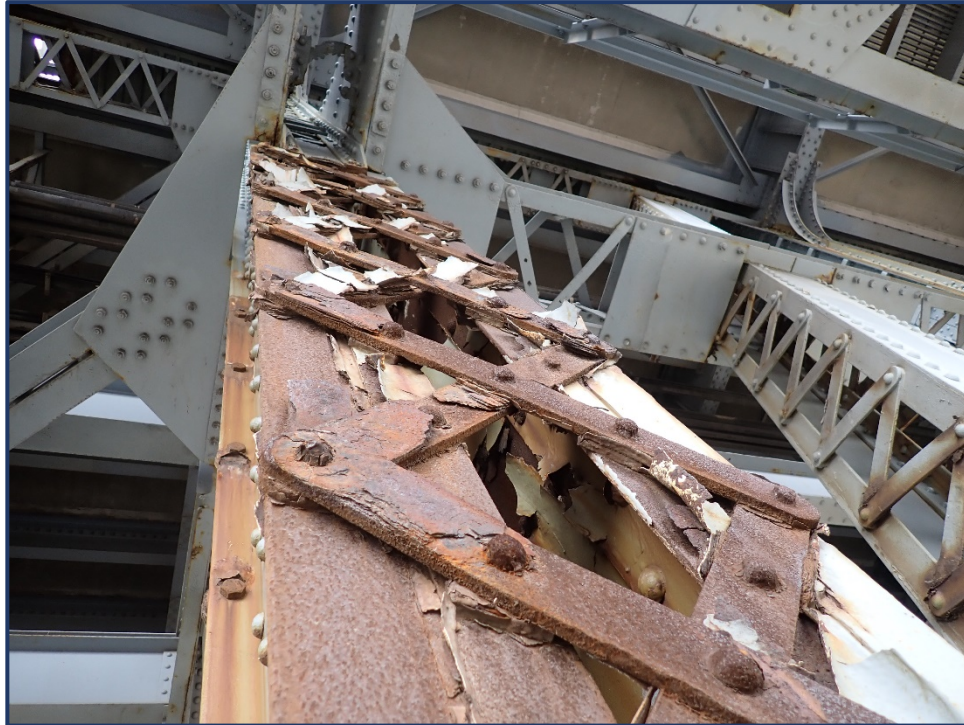
Photo 120-3 – Span 4, South Truss, U2”-L2’, Active Corrosion extending down from Upper Deck
