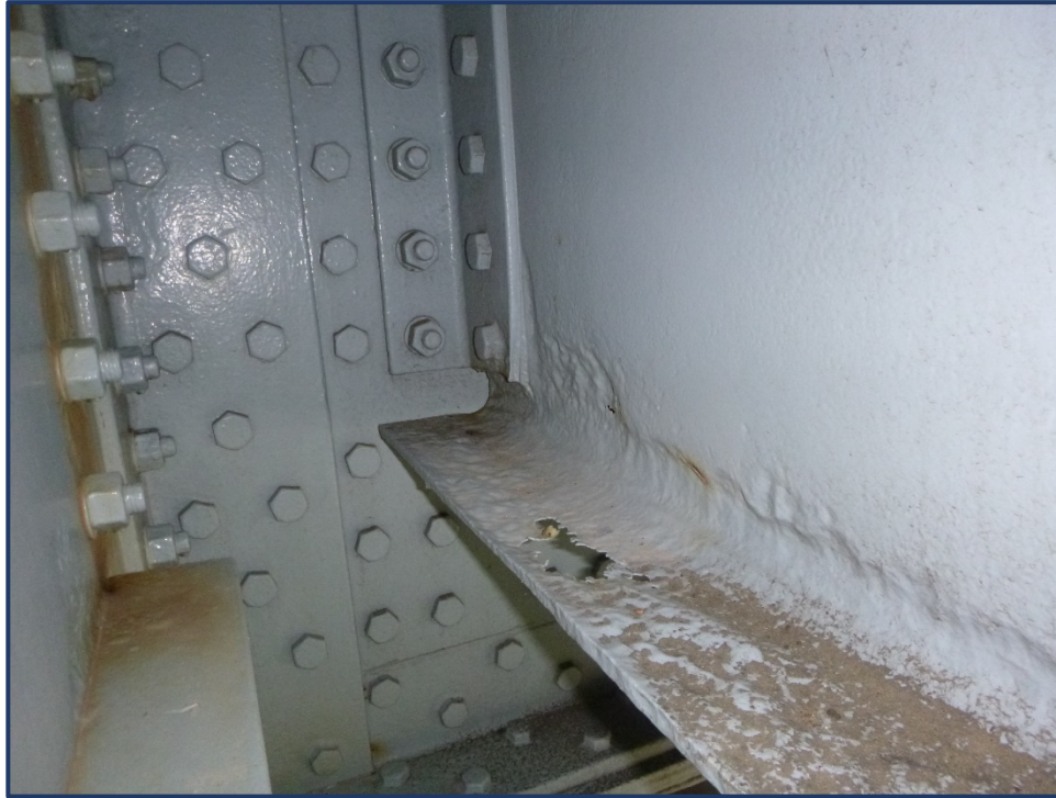
Photo 113-1 – Span 4, Upper Deck Stinger E, Bay 2-3, Painted over Section Loss and Hole in Bottom Flange at FB3
