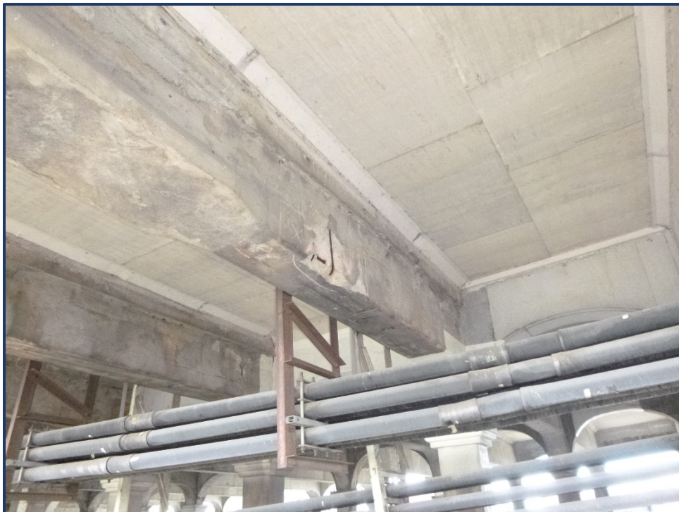
Photo 155-4 – Span 3, Upper Deck FB 11, South Bay, Spalling and Delamination
