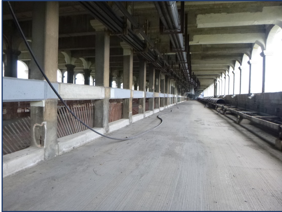
Photo UT-1 – Sagging Utility Line on Maintenance Deck
