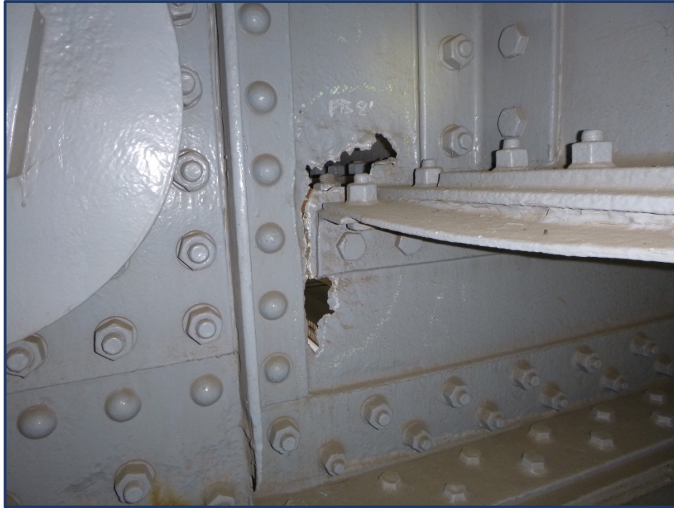
Photo 152-2 – Span 4, Upper FB8', Corrosion Holes in Web, N. of Stringer E
