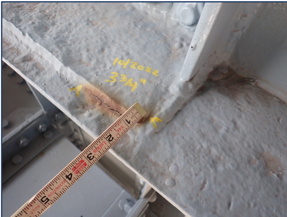
Photo 152-5 – Span 4, Lower FB9', North End, West Face, Crack in Top Flange Stiffener Retrofit
