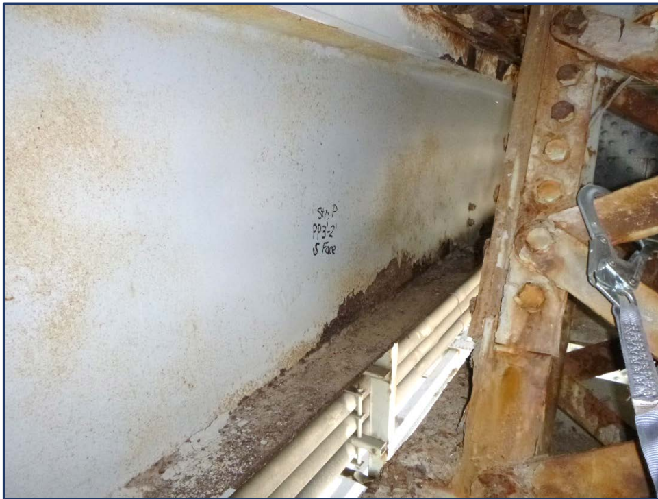
Photo 113-3 – Span 4, Upper Deck Stinger P, Bay 3'-2', Active Section Loss with Small Holes in Bottom Flange
