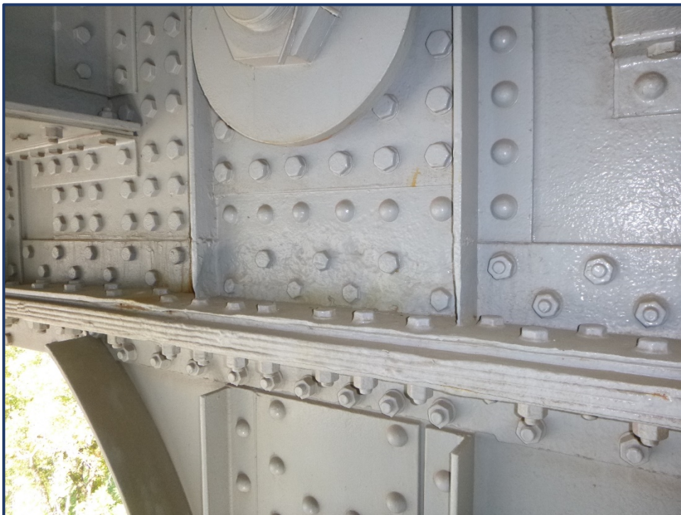
Photo 152-1 – Span 4, Upper FBs, Typical Painted over Pitting and Pack Rust at Deck Opening
