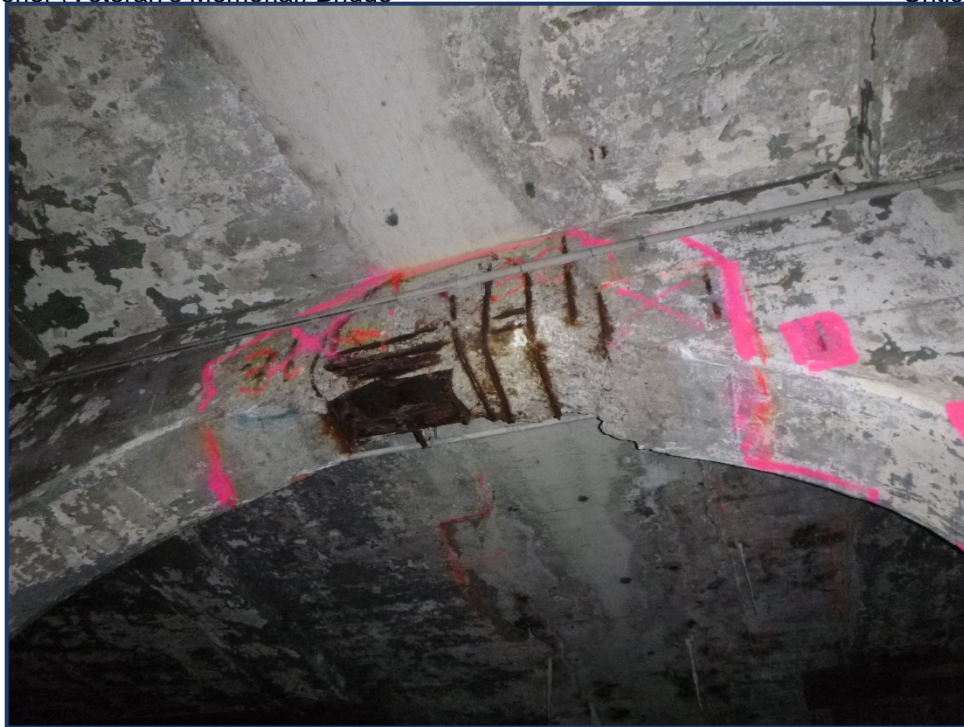
Photo 110-1 – West Station, Spalling of Concrete Beam
