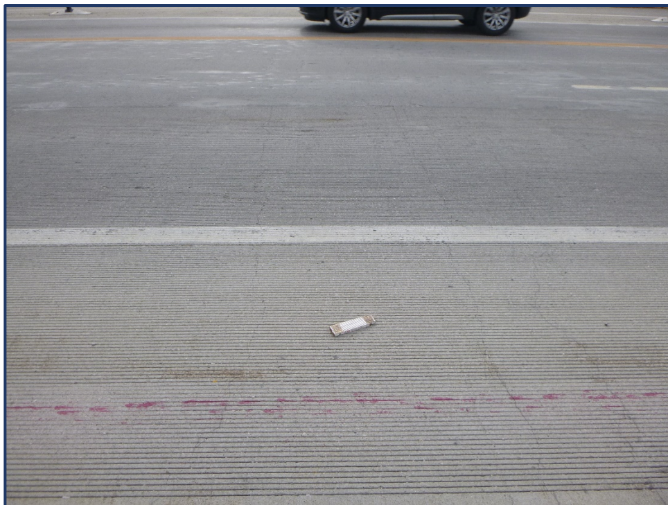
Photo 510-1 – Map Cracking in Wearing Surface
