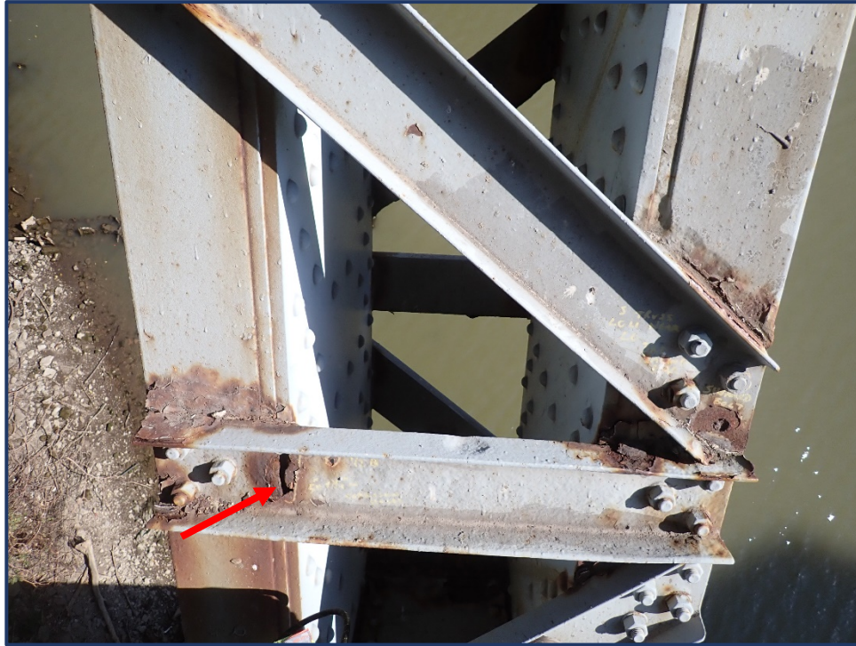
Photo 120-5 – Span 4, South Truss, L0-L1, Active Section Loss and Corrosion Hole in Lacing Bar
