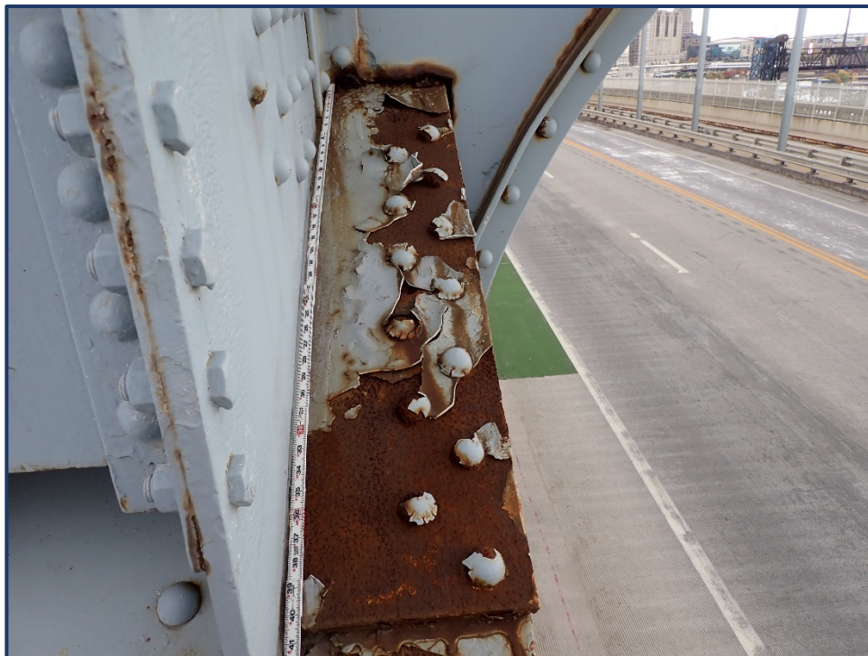
Photo 120-4 – Span 4, North Truss, L5-L6, Active Corrosion at Lateral Bracing
