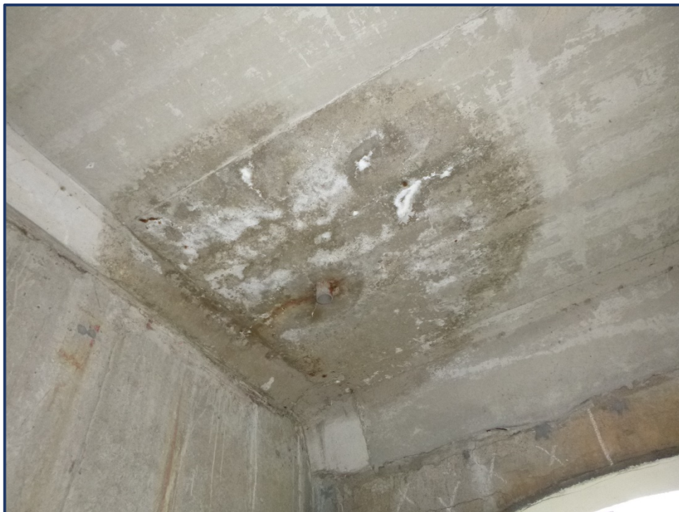
Photo 12-4 – Main Spans, Deck Saturation with Mottling and Efflorescence
