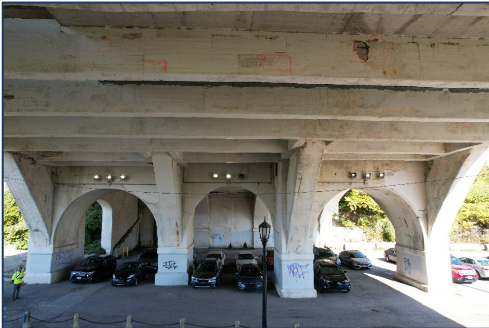
Photo 155-2 – Span 12, Widespread Cracking, Delamination and Spalling of Lower Deck Floorbeams
