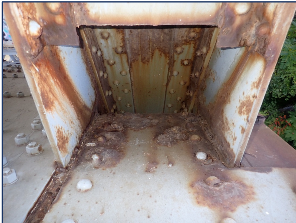
Photo 162-1 – Span 4, North Truss, L1 Gusset Plates, Active Pitting along L1-L2
