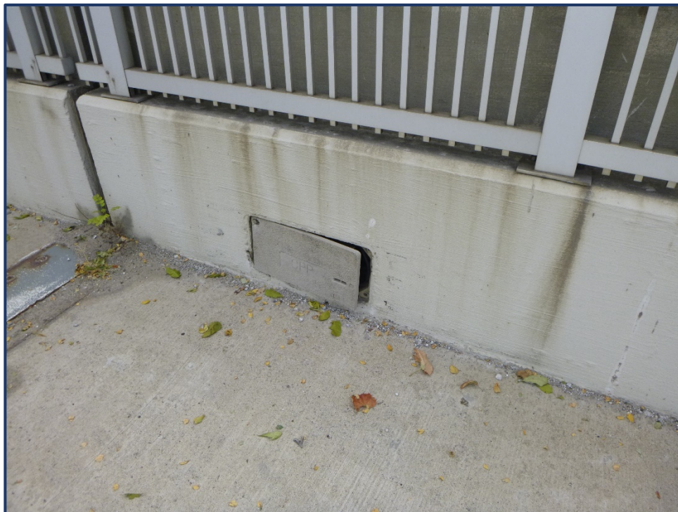
Photo UT-2 – Partially Detached Electric Junction Box Cover, South Railing, Span 1A
