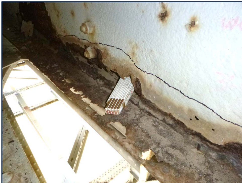
Photo 113-2 – Span 4, Upper Deck Stinger P, Bay 4'-3', Active Section Loss with Holes in Web and Bottom Flange
