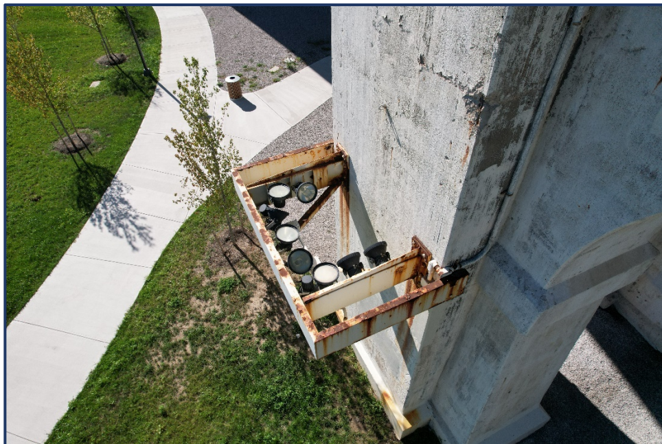
Photo UT-4 – Typical Corrosion and Minor Section Loss on Tower Light Brackets
