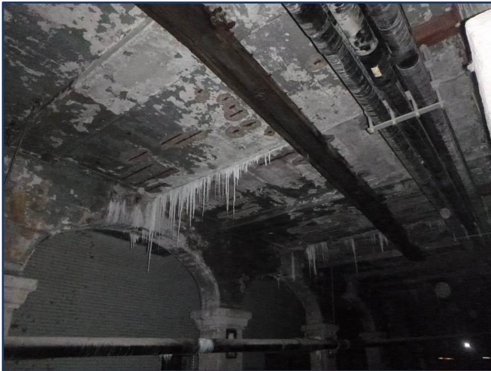
Photo 12-2 – West Station, Typical Scattered Deck Spalling with Saturation and Efflorescence
