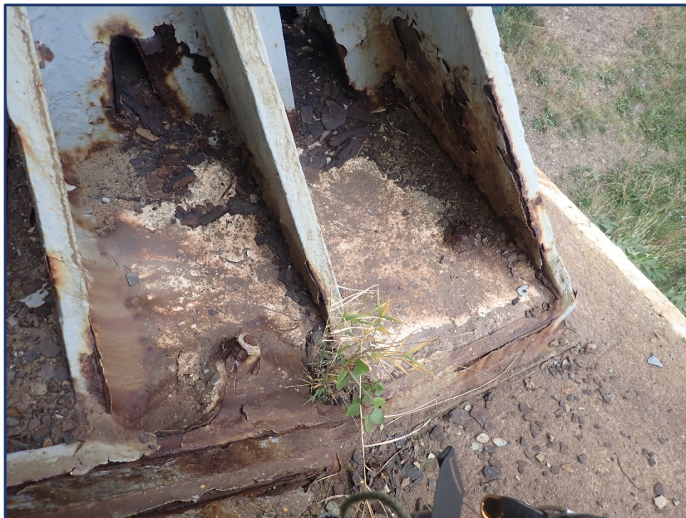
Photo 313-4 – Span 4, North Truss, L0' Bearing, Anchor Bolt & Nut Section Loss
