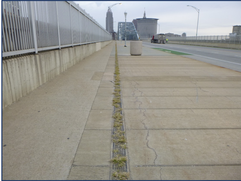
Photo 815-3 – North Sidewalk Longitudinal Drain, Typical Clogging with Debris and Vegetation Growth
