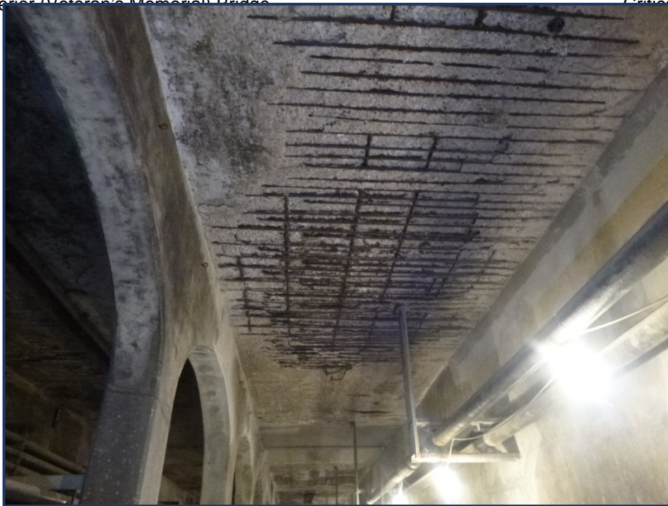
Photo 12-1 – Detroit Ave Tunnel, Typical Spalling of Non-structural Deck
