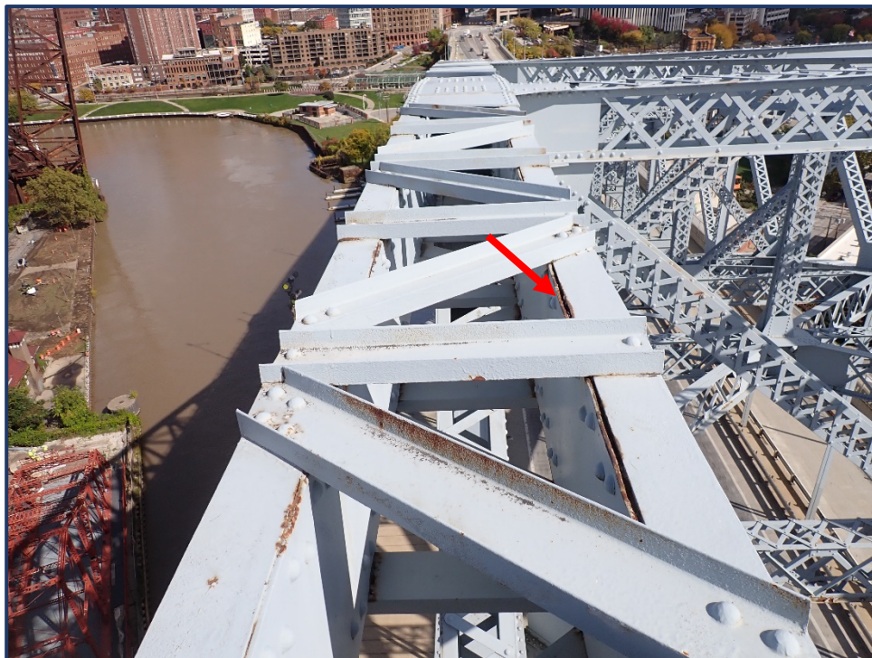
Photo 120-2 – Span 4, North Truss, U12-U11', Active Pack Rust between Web Plate and Flange Angles.
