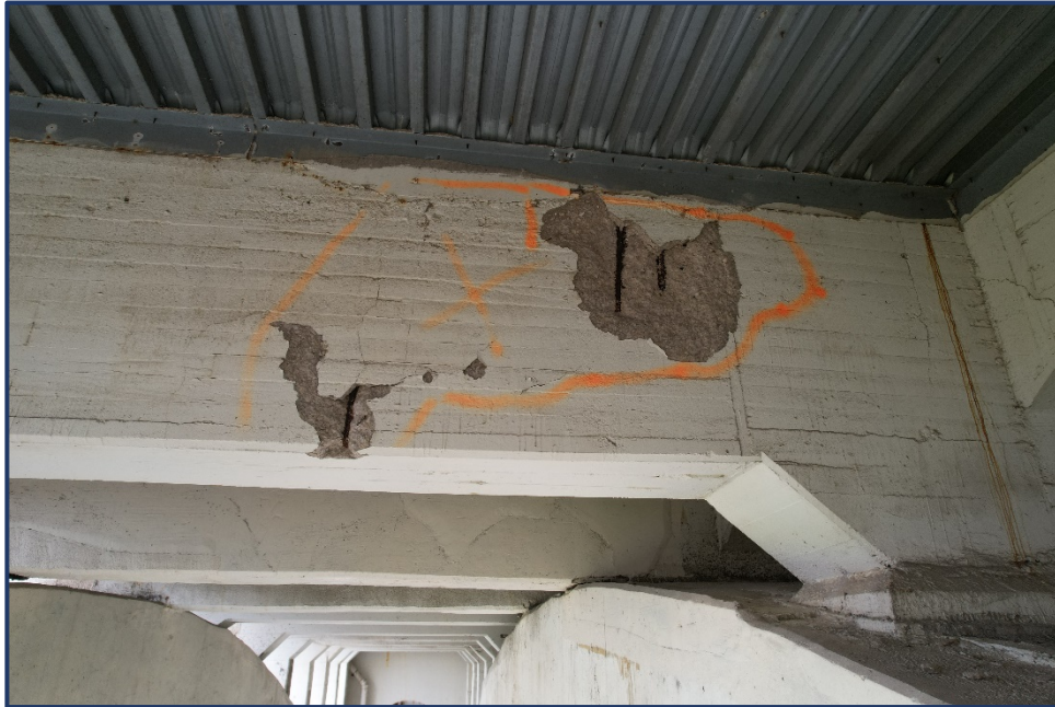
Photo 155-1 – Span 2, Lower Deck Floorbeam, South Bay, Delamination and Spalling with Exposed Reinforcing
