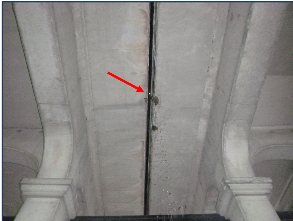
Photo 300-3 – Pier 10 Joint, Section of Seal Tearing
