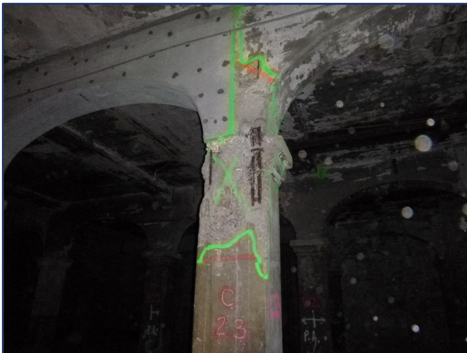
Photo 205-4 – West Station, Column Spalling with Exposed Reinforcing
