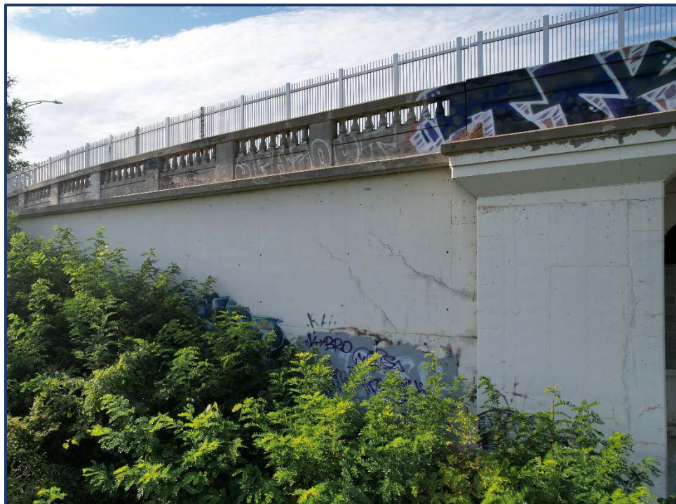
Photo WW-1 – West Abutment South Wingwall, Areas of Cracking
