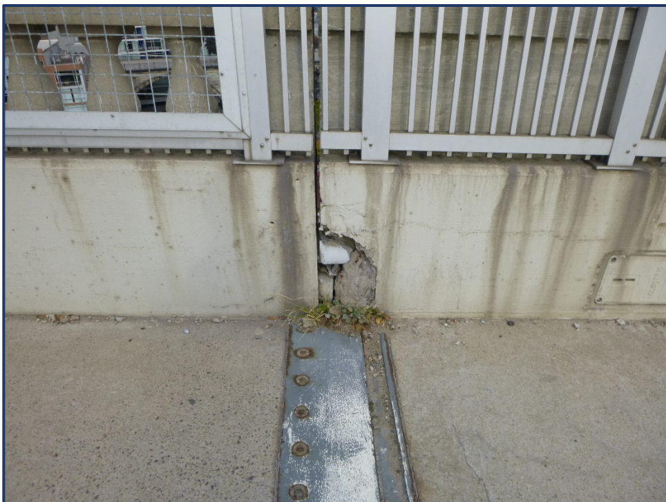
Photo 331-1 – South Rail, Typical Spalling at Deck Joints
