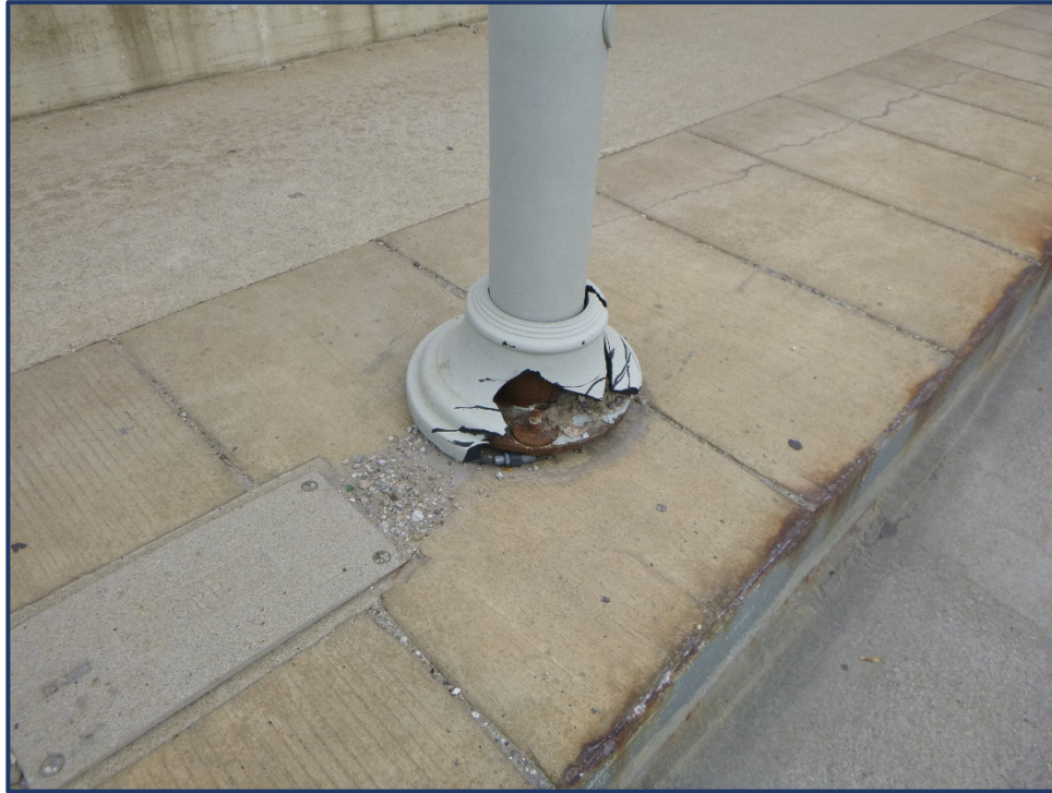
Photo UT-3 – Broken Light Pole Base Cover on North Sidewalk
