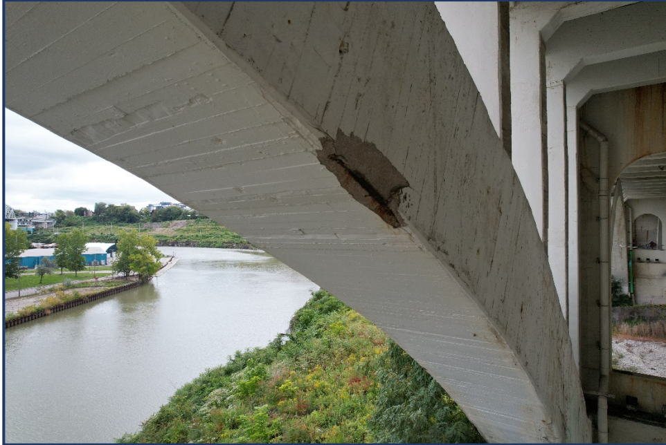
Photo 144-4 – Span 3, South Exterior Arch, Spall with Exposed Reinforcing
