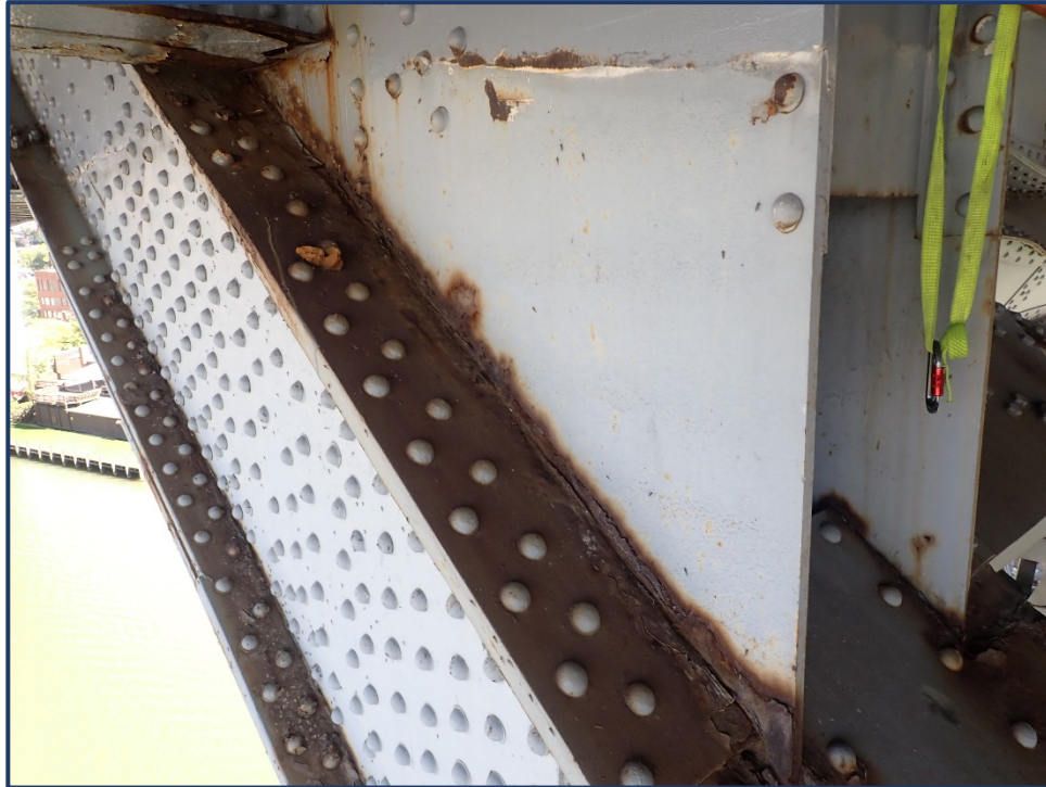
Photo 162-2 – Span 4, North Truss, L3 South Gusset Plate, Active Pitting & Pack Rust
