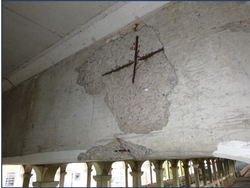
Photo 155-3 – Span 3, Upper Deck FB 3, Center Bay, Spalling and Delamination
