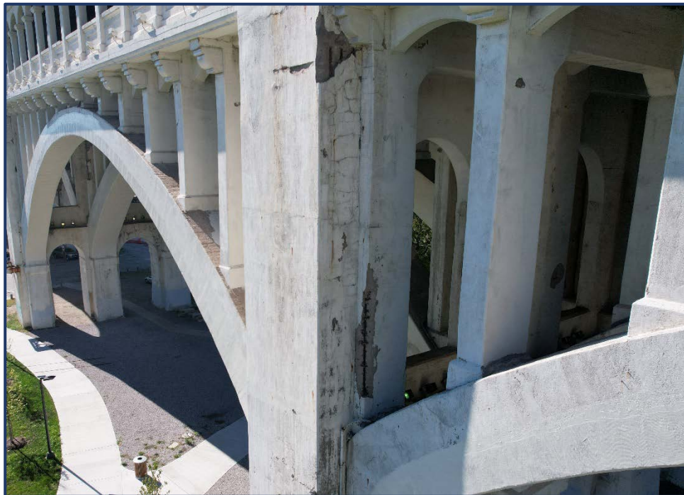
Photo 205-5 – Pier 10, South Tower, Widespread Delamination and Spalling with Exposed Reinforcing
