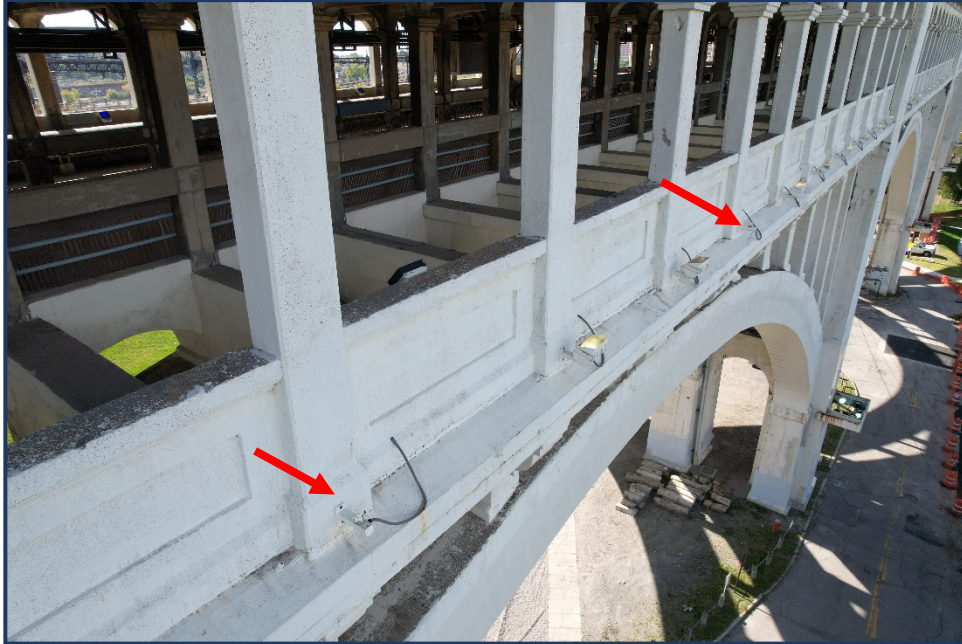
Photo UT-5 – Broken Architectural Lights, Span 8 North Fascia
