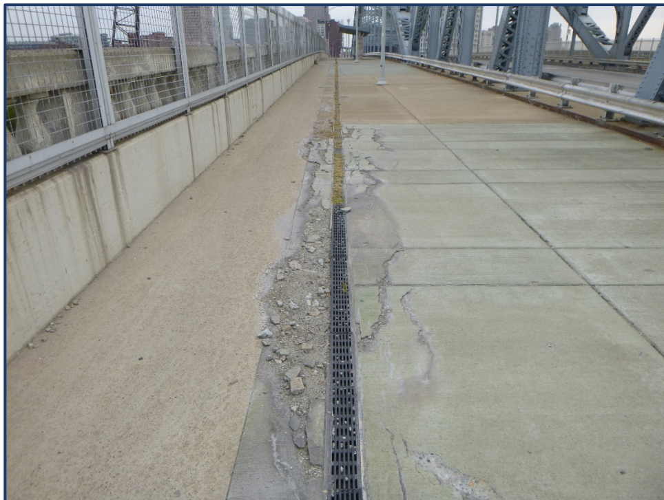
Photo CS-2 – Span 4 North Sidewalk, Spalling, Delamination and Cracking along Longitudinal Drain
