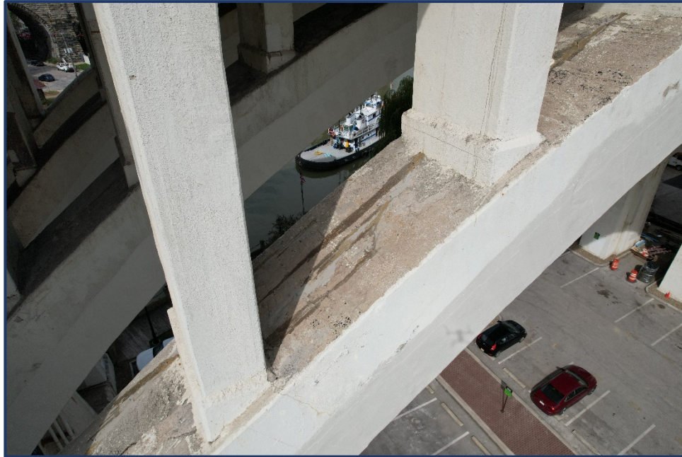
Photo 144-2 – Span 5, South Exterior Arch, Sealed Cracks on Top of Arch, with FRP on Underside
