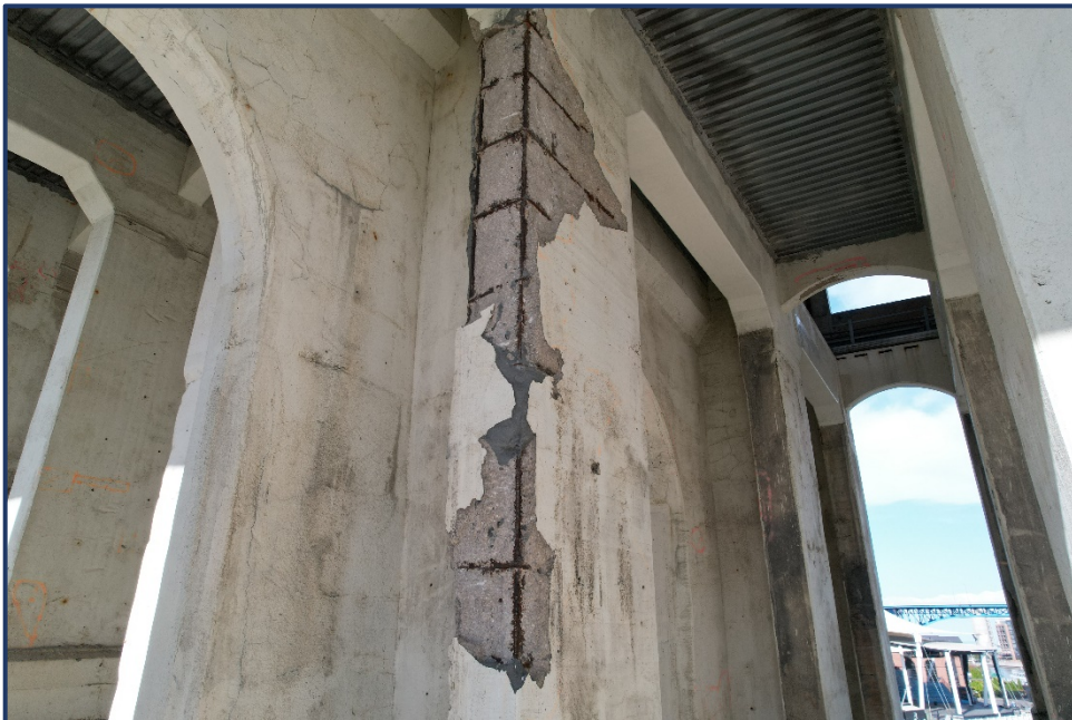
Photo 144-5 – Span 8, South Interior Arch, Spalling with Exposed Reinforcing of Arch Column
