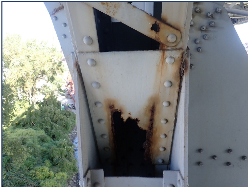
Photo 120-6 – Span 4, North Truss, U1-L2, Perforations in Batten Plate, with Reactivating Corrosion
