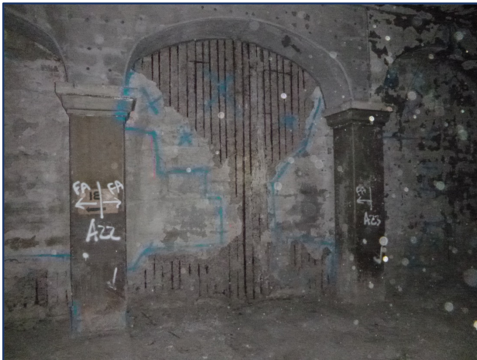
Photo 215-1 – West Station, Spalling with Exposed Reinforcing on Walls
