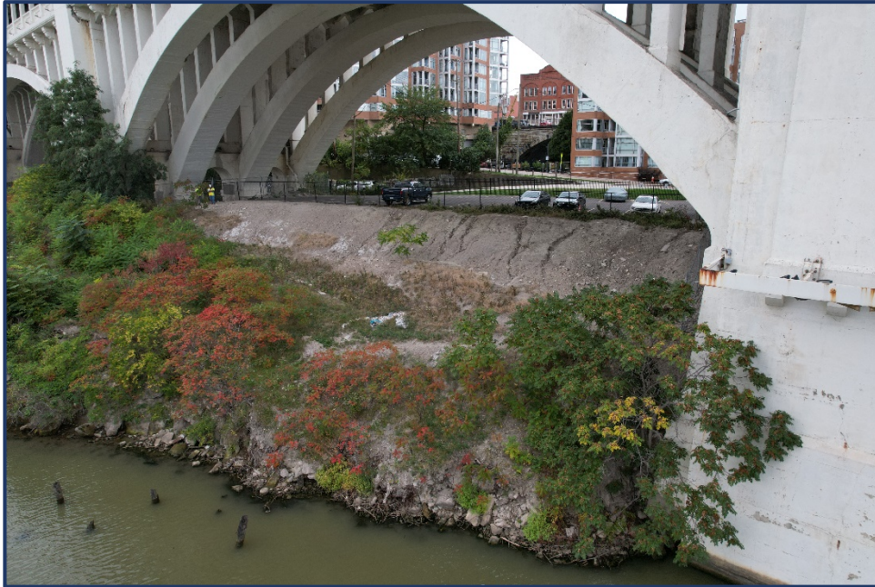
Photo APR-1 – Erosion of Embankment on South Side Span 3
