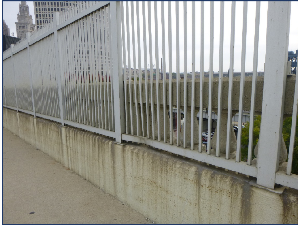
Photo 331-2 – South Rail Fence, Area of Damage
