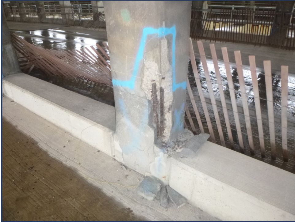
Photo 144-6 – Span 6, South Interior Arch, Spalling of Arch Column
