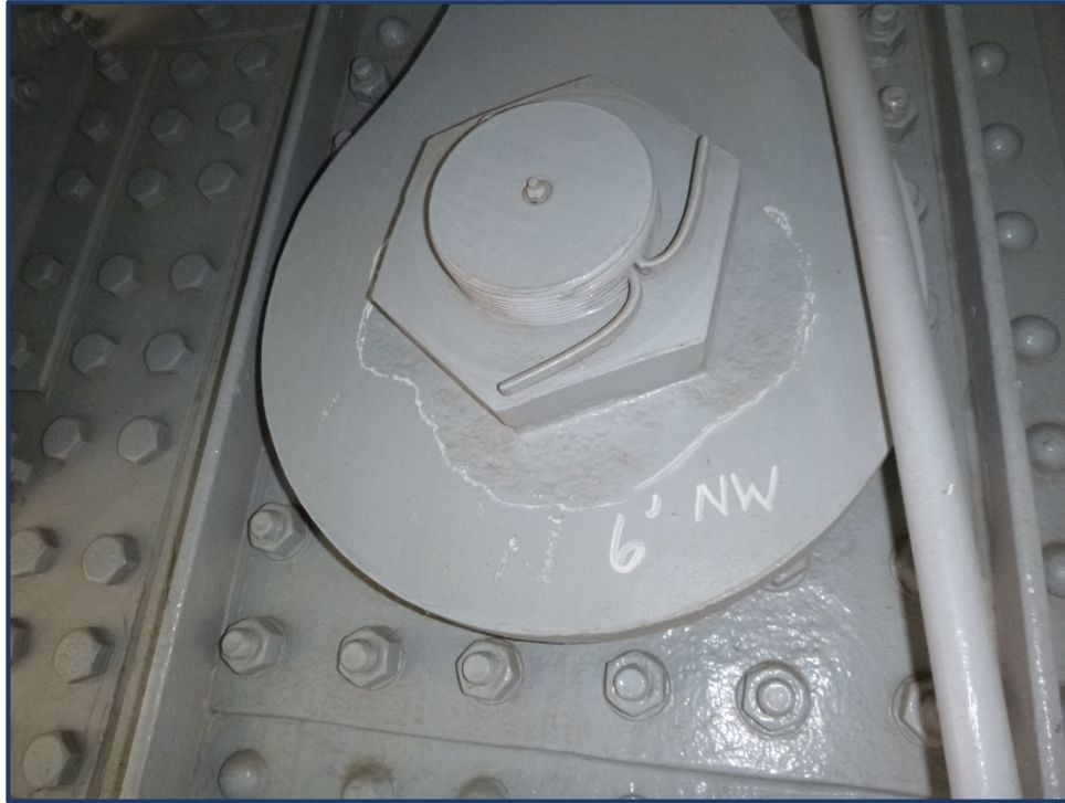
Photo 161-1 – Span 4, North Truss, Hanger Connection at Upper FB8', Painted over Pitting around Pin
