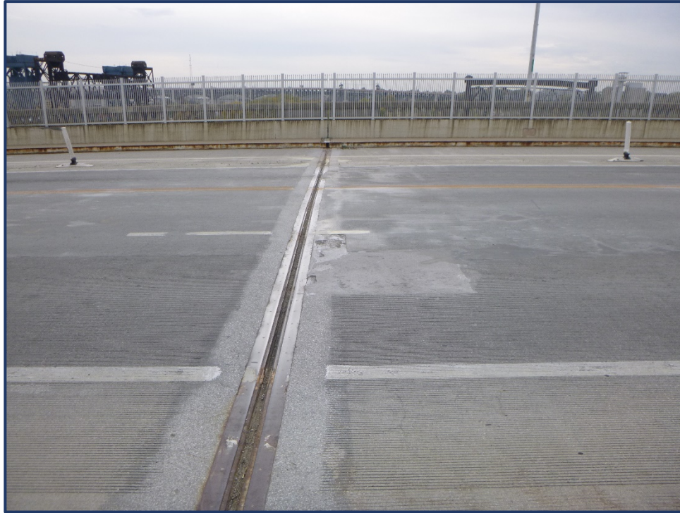
Photo 510-2 – Area of Concrete Patching in Wearing Surface
