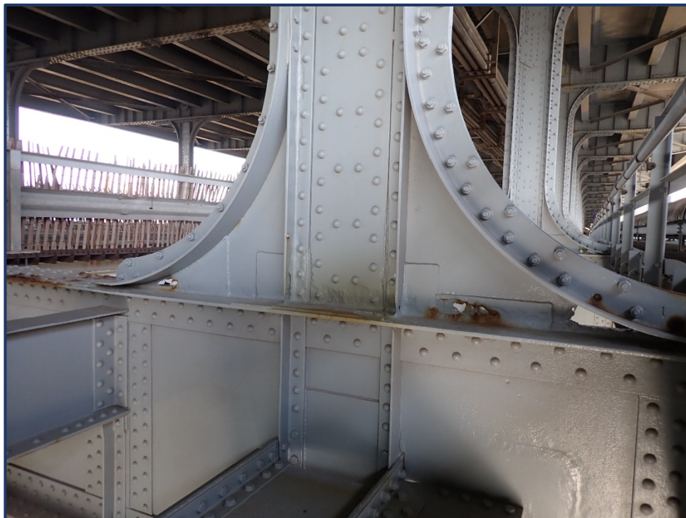
Photo 152-3 – Span 4, Lower FB10 at South Truss, Reactivating Painted Over Section Loss in Top Flange and Stiffeners
