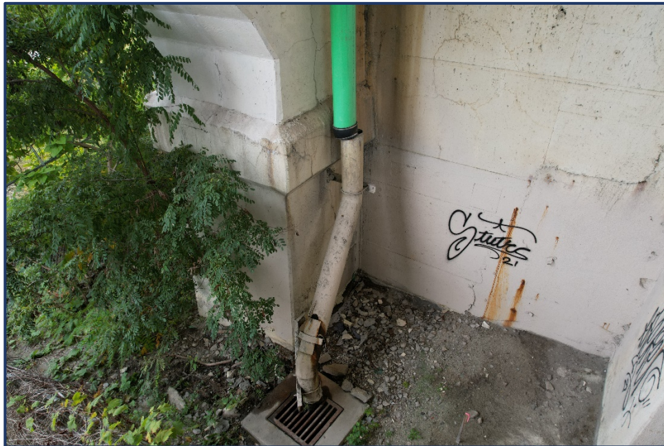
Photo 815-1 – Pier 1, East Face, South Downspout Fully Clogged at Catch Basin and Disconnected at Outlet Section
