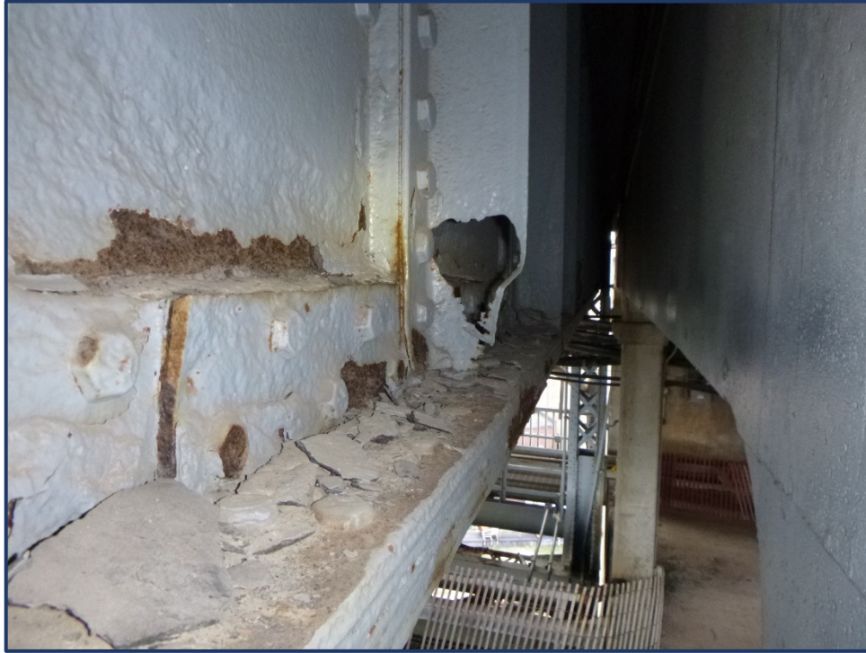
Photo 152-4 – Span 4, Upper FB0, Painted over Pitting, and Perforations to Transverse Stiffeners
