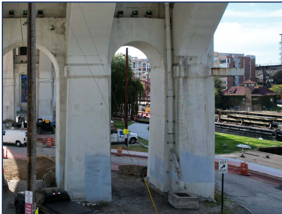
Photo 205-2 – Pier 6, East Face, Cracking of North Column
