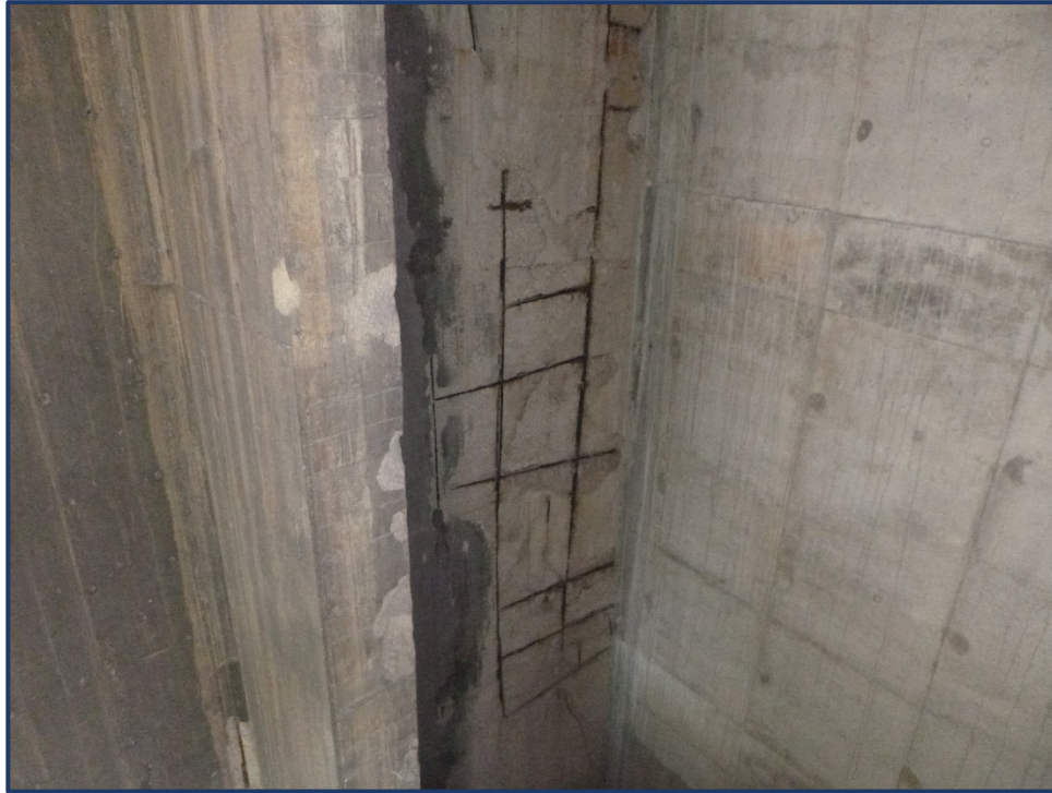
Photo 210-3 – Pier 4, Typical Spalling of Interior Face of Pier Walls
