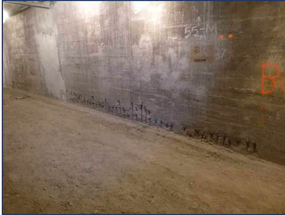
Photo 215-2 – Detroit Ave. Tunnel, Typical Spalling on Lower Portions of Walls
