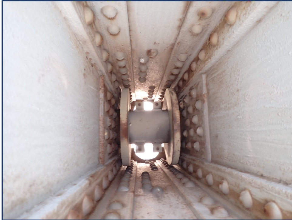
Photo 120-7– Span 4, South Truss, L11, Reactivating Pitting around Hanger Pin
