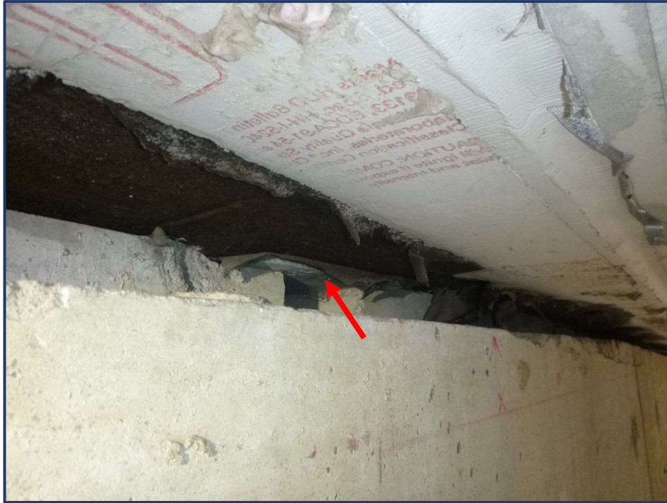
Photo 313-5 – Pier 11, Slab/Floorbeam Bearing Plates between Ribs B & C, Shifting/Missing Bearing Plates
