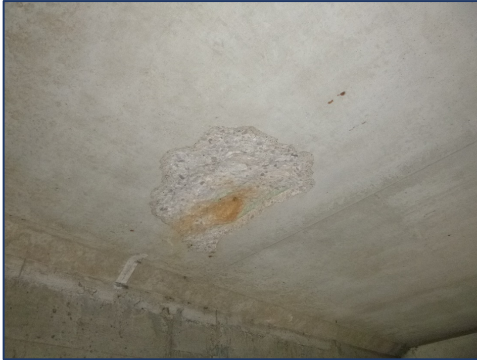
Photo 12-3 – Main Spans, Typical Scattered Deck Spalling with Exposed Reinforcing
