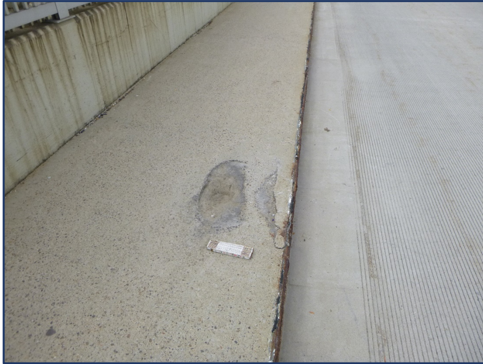
Photo CS-1 – South Sidewalk, Typical Edge Spalling
