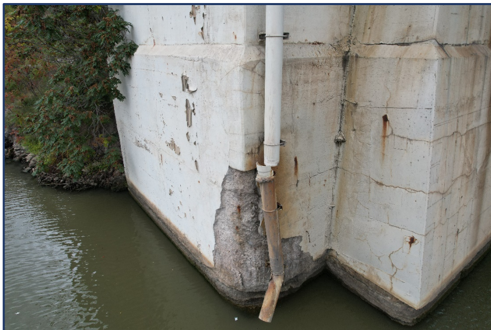
Photo 815-2 – Pier 3, South Downspout Disconnected at Outlet
