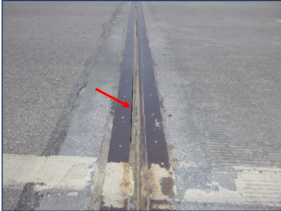
Photo 300-4 Joint 1A, Section of Broken Intermittent Fillet Welds in Joint Armor
