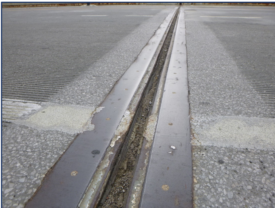
Photo 300-1 – Joint 8, Debris Impaction and Section of Seal Pulling out of Retainer
