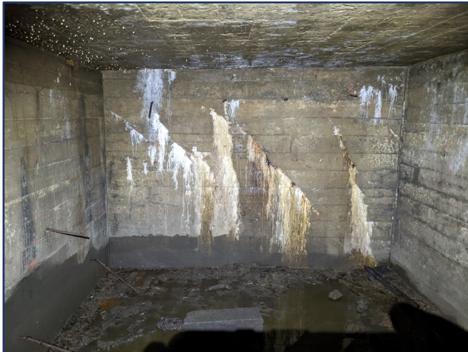
Photo AC-1 – West Abutment Chamber, Typical Cracking with Efflorescence
