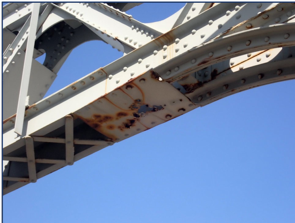
Photo BR-1 – Active Corrosion and Pack Rust on Sway Bracing Members
