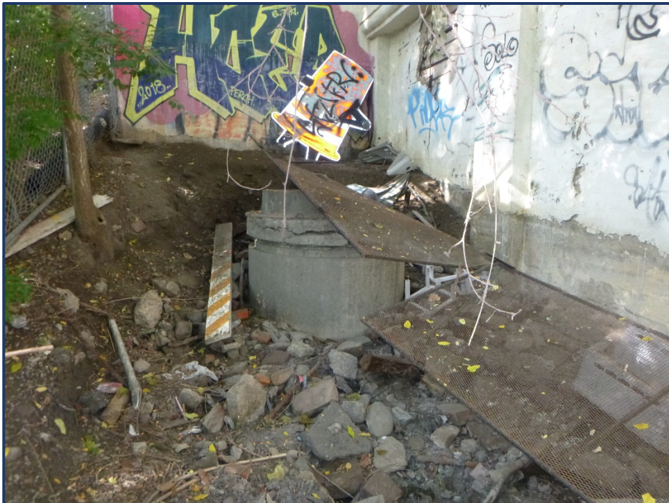
Photo APR-6 – Failed Preventive Access Steel Mesh on South Side of Span 1A
