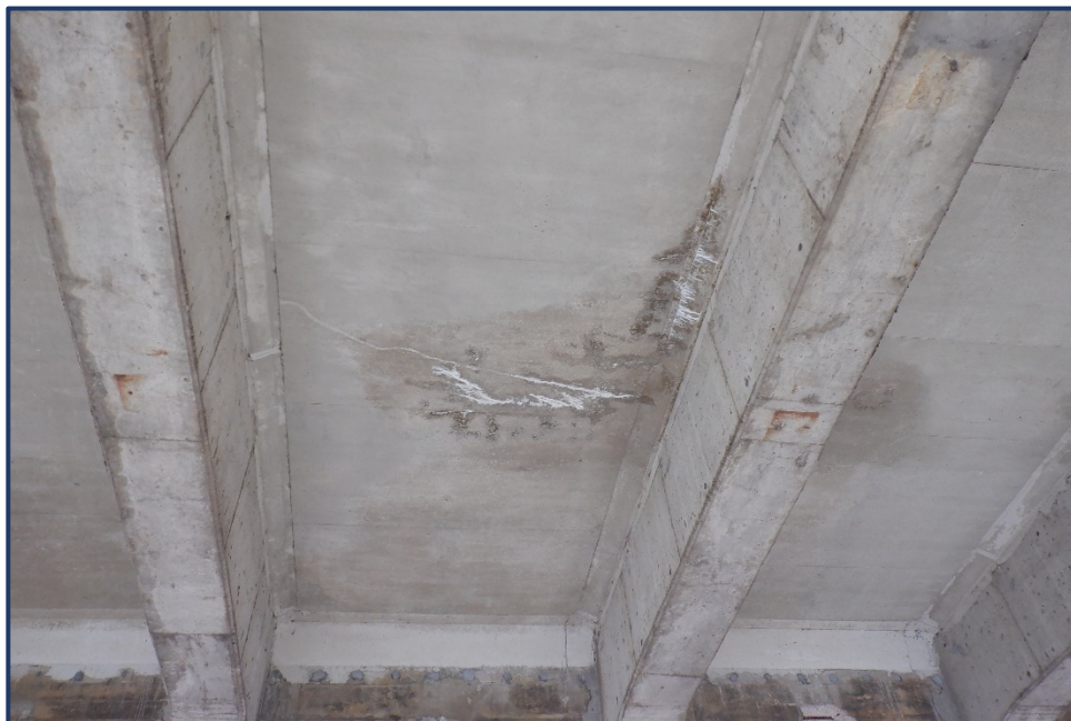
Photo 12-4 – Main Spans, Deck Saturation with Mottling and Efflorescence
