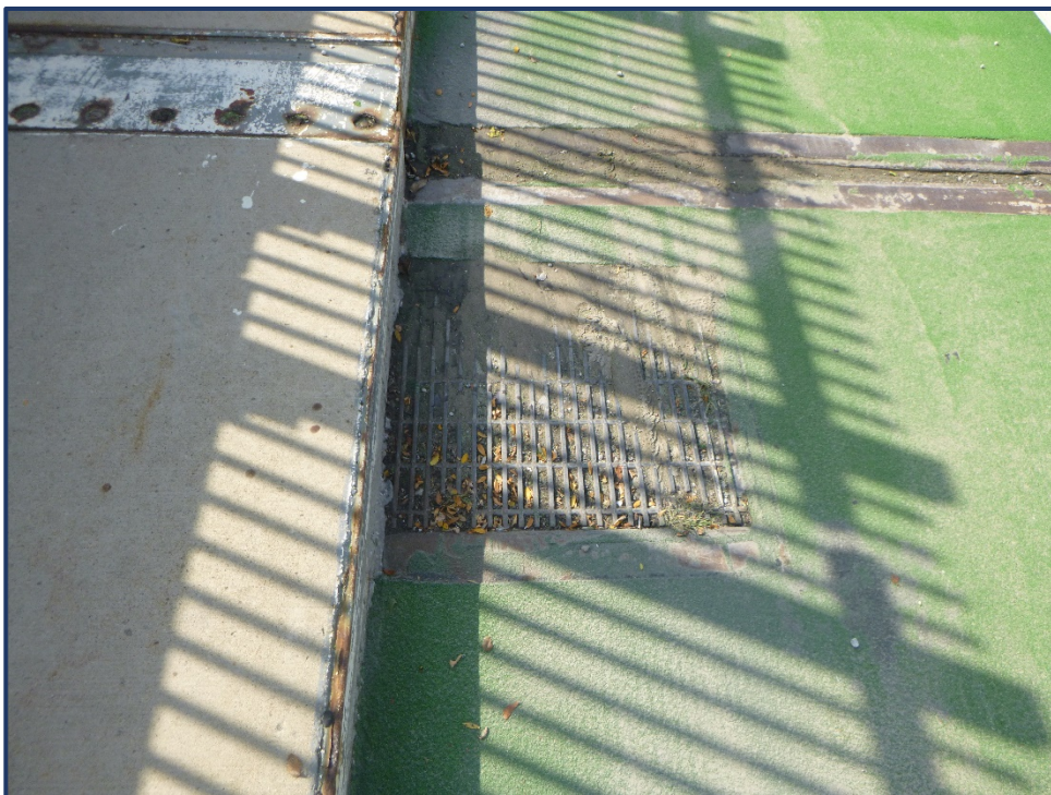
Photo 815-4 – Span 1, South Curb Scupper Inlet Fully Clogged with Debris
