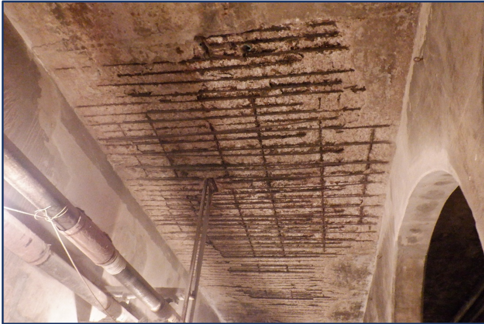
Photo 12-1 – Detroit Ave Tunnel, Typical Spalling of Non-structural Deck
