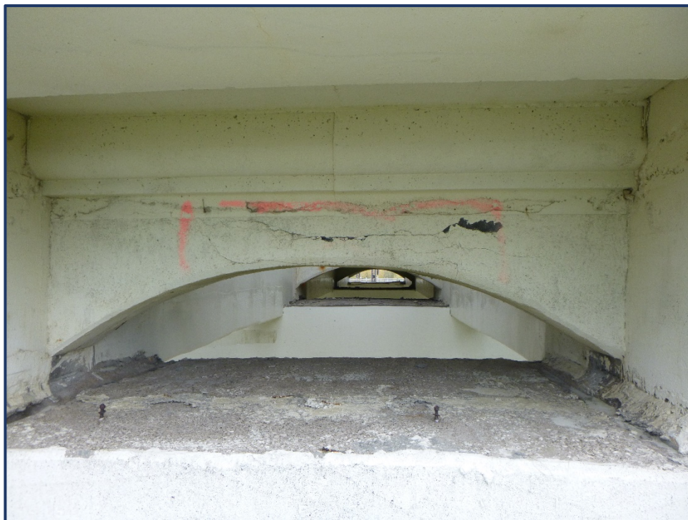
Photo 144-7 – Span 8, North Exterior Arch, Cracking and Delamination of Jack Arch
