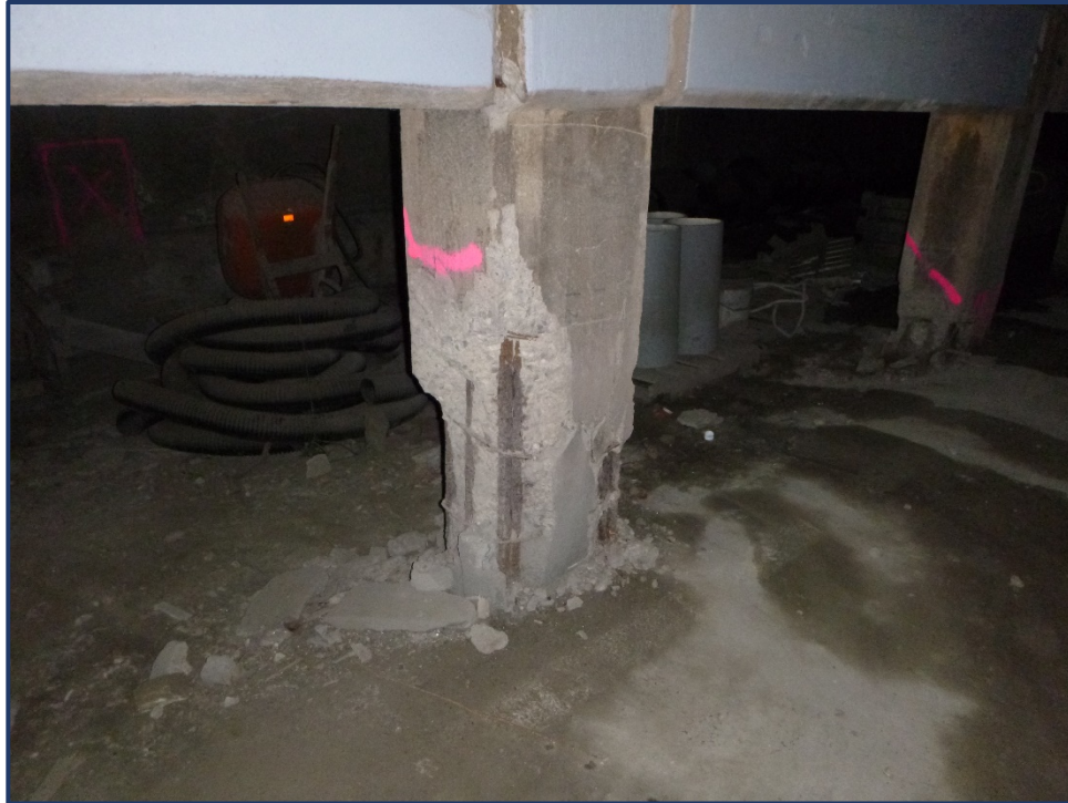
Photo 205-3 – Span 1A, Typical Column Spalling with Exposed Reinforcing
