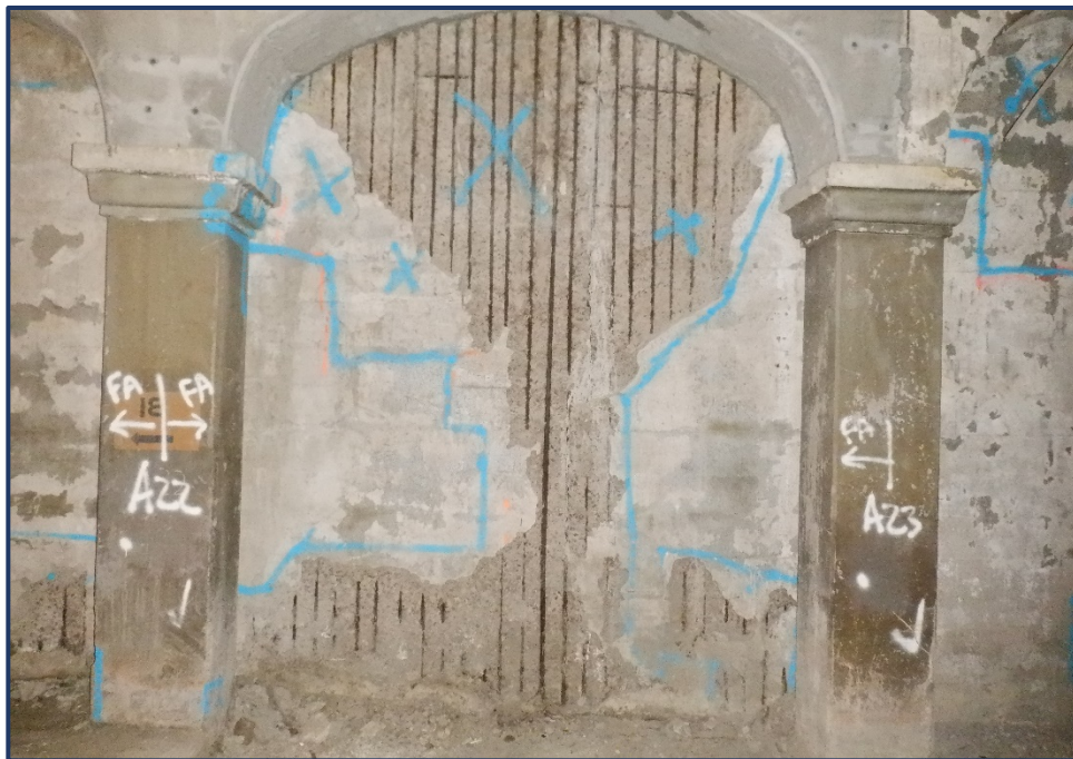
Photo 215-1 – West Station, Spalling with Exposed Reinforcing on Walls
