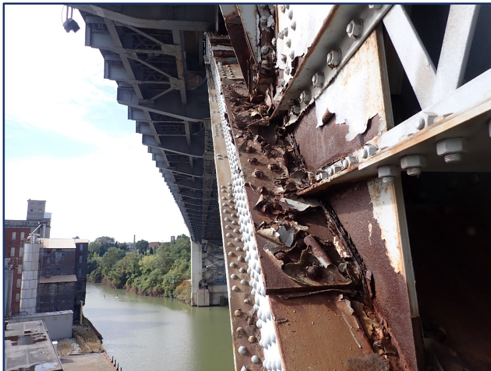
Photo 120-3 – Span 4, South Truss, L2'-L3", Active Corrosion and Pack Rust
