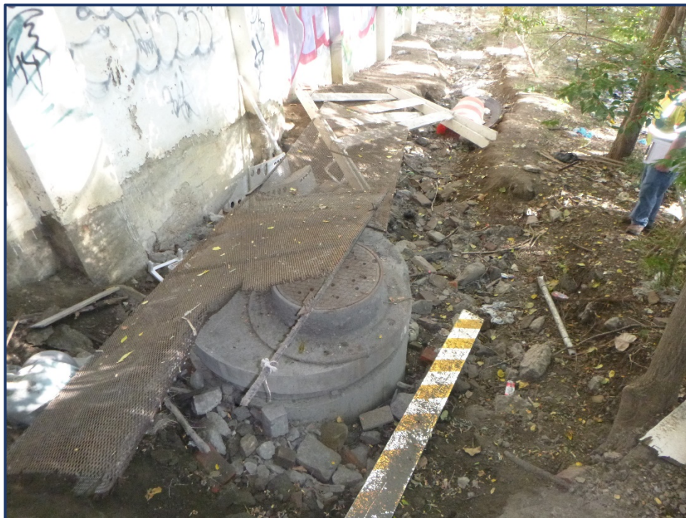
Photo APR-2 – Erosion Hole and Channel on South Side of Span 1A
