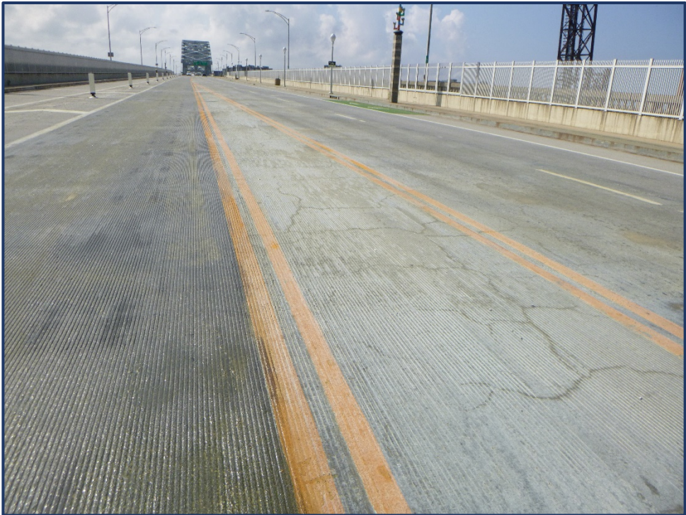
Photo 510-1 – Map Cracking in Wearing Surface
