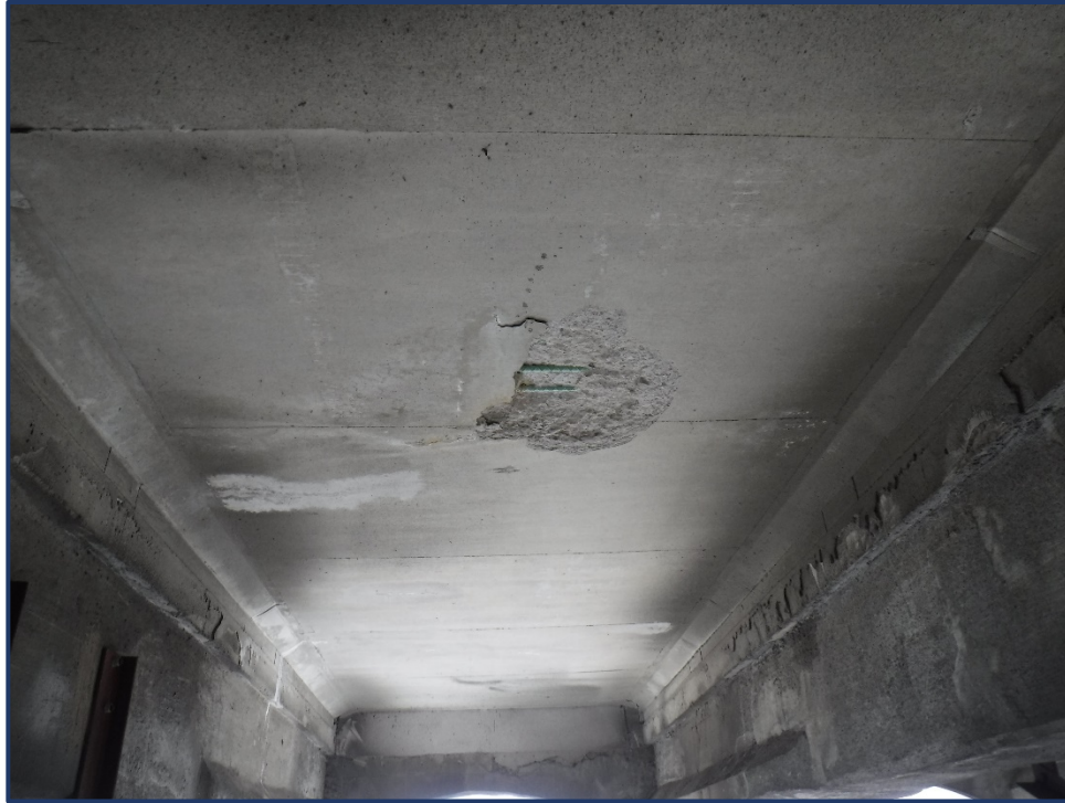
Photo 12-3 – Main Spans, Typical Scattered Deck Spalling
