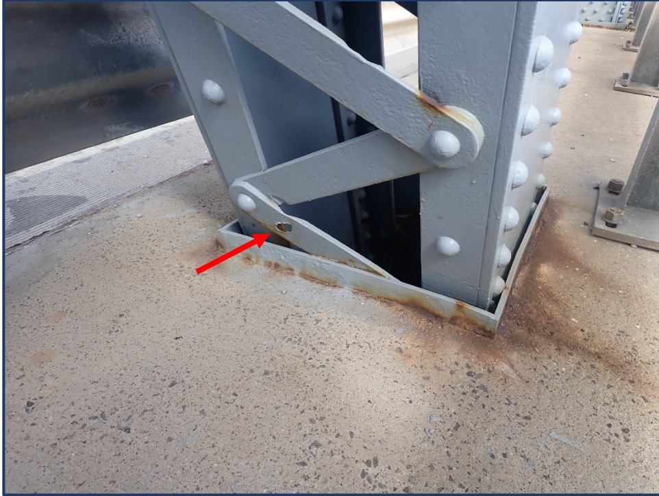
Photo 120-4 – Span 4, South Truss, U1-L1, Painted Over Section Loss and Corrosion Hole in Lacing Bar at Deck Level
