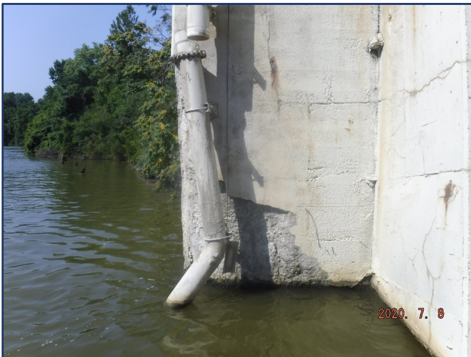
Photo 815-2 – Pier 3, South Downspout Disconnected at Outlet
