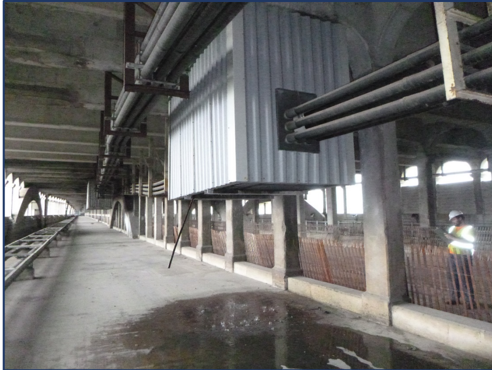
Photo 815-5 – Span 13, Heavy Deck Drainage through Utility Manhole
