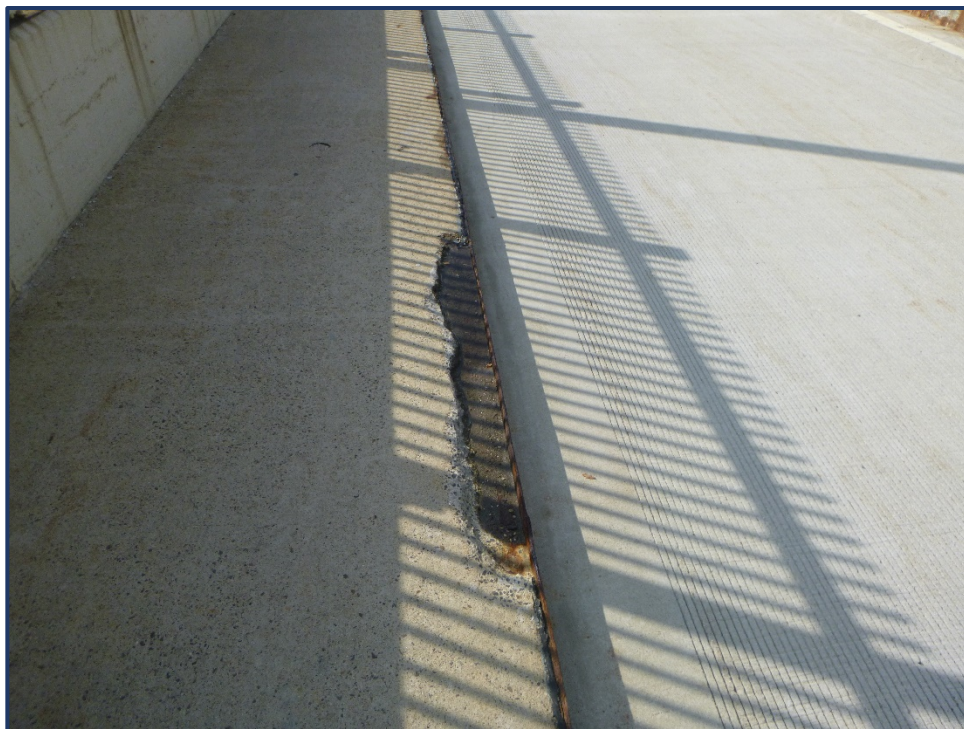
Photo CS-1 – South Sidewalk, Typical Edge Spalling
