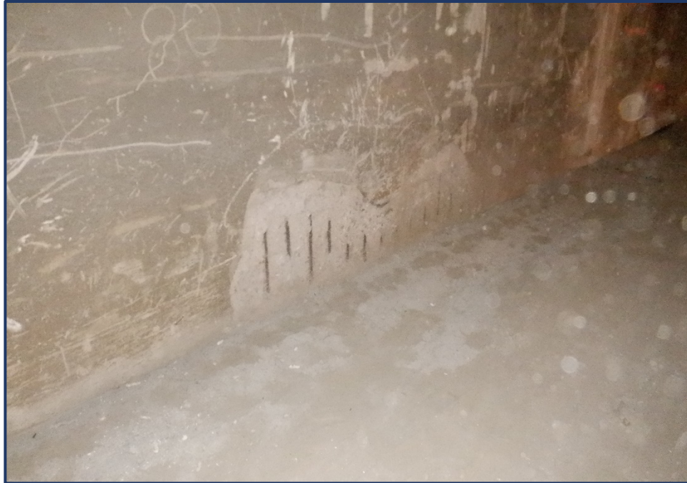
Photo 215-2 – Detroit Ave. Tunnel, Typical Spalling on Lower Portions of Walls
