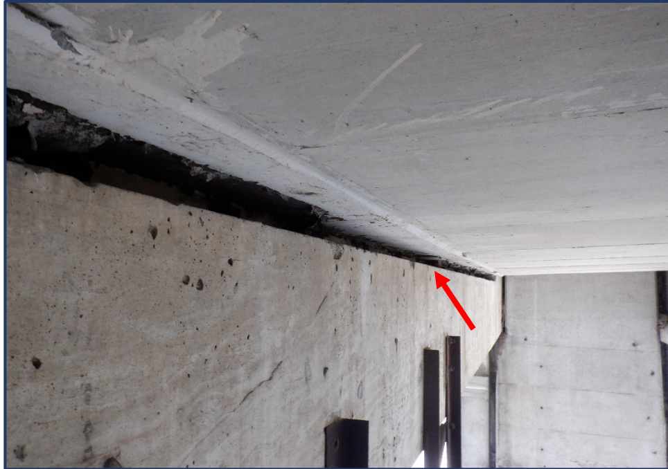
Photo 313-5 – Pier 11, Slab/Floorbeam Bearing Plates between Ribs C & D, Movement of Bearing Plates
