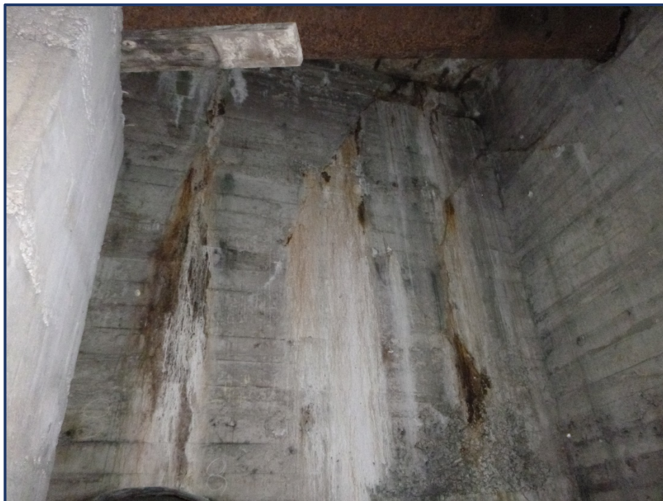
Photo AC-1 – West Abutment Chamber, Typical Cracking with Staining and Shallow Spalling
