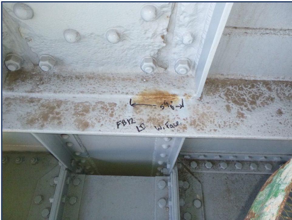
Photo 152-5 – Span 4, Lower FB12, North End, West Face, 5-5/8" Crack in Top Flange Stiffener Retrofit
