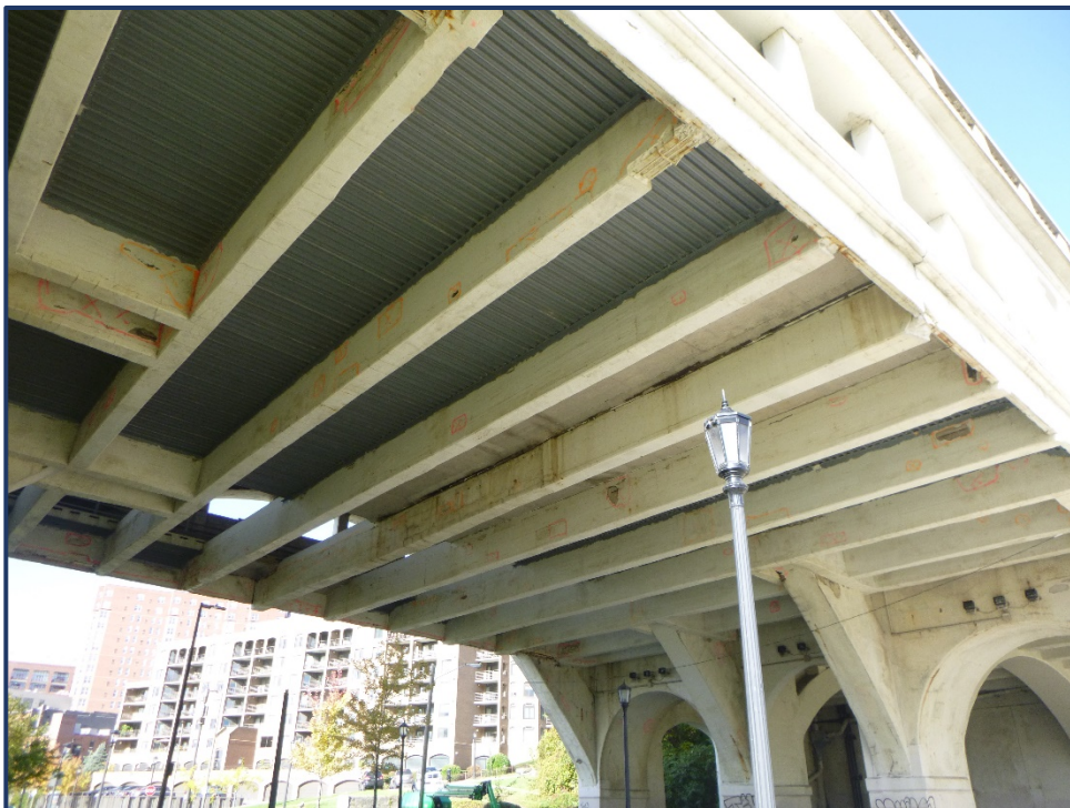
Photo 155-2 – Span 12, Widespread Cracking, Delamination and Spalling of Lower Deck Floorbeams
