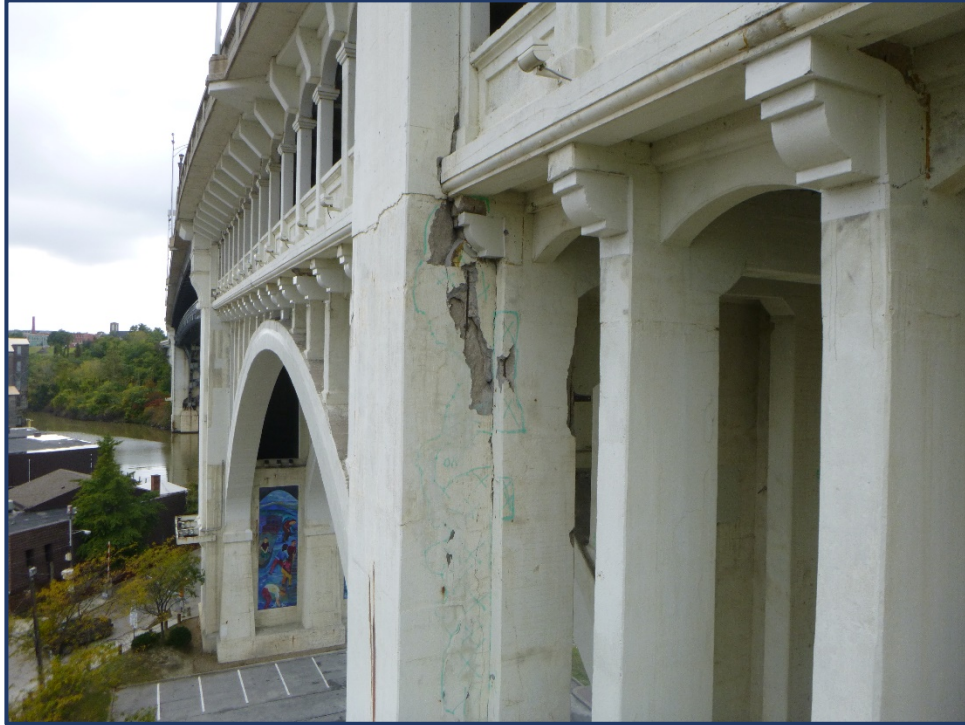
Photo 205-5 – Pier 5, South Tower, Widespread Delamination and Spalling with Exposed Reinforcing
