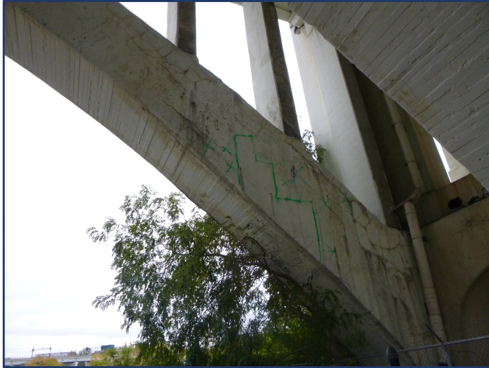
Photo 144-4 – Span 3, South Exterior Arch, Map Cracking and Delamination of Arch Rib
