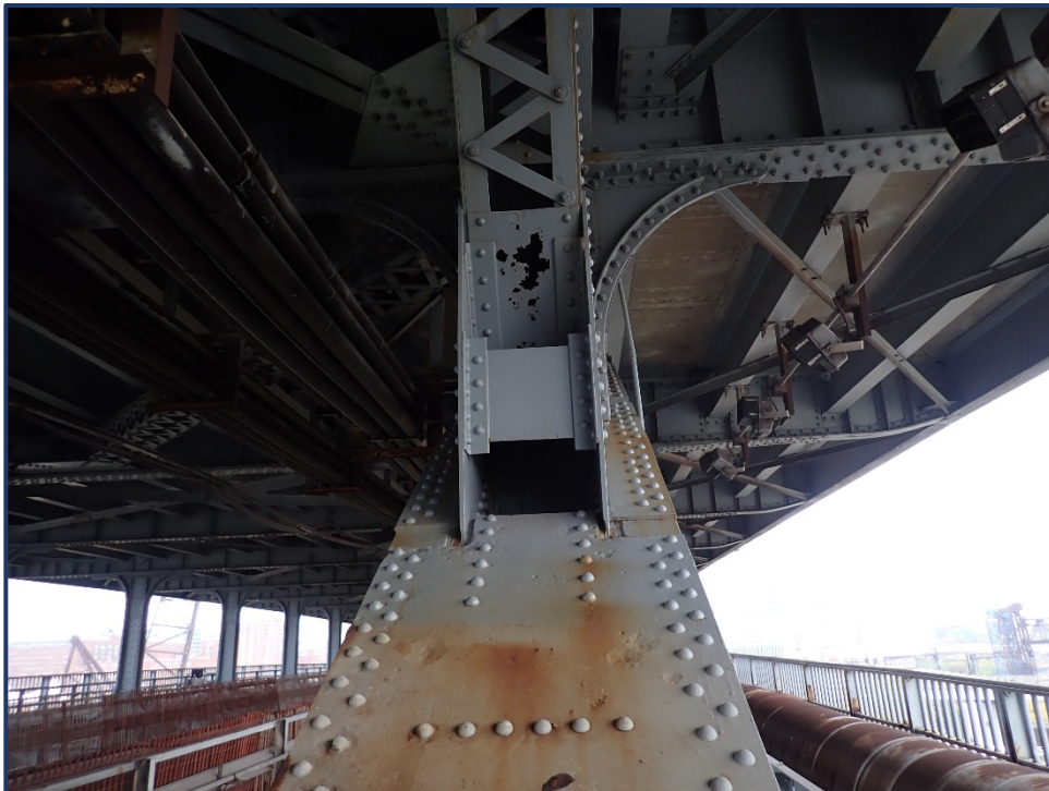
Photo 120-5 – Span 4, South Truss, U3-L4,, Perforations in Batten Plate, with Reactivating Corrosion
