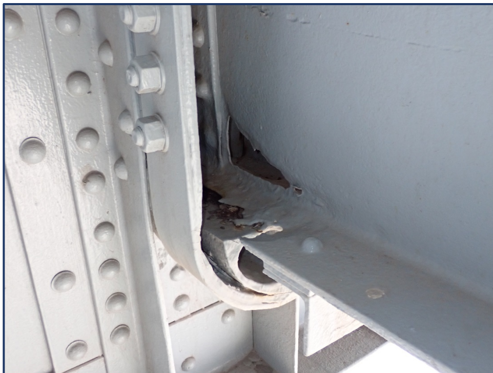
Photo 113-4 – Span 4, Lower Deck Stringer K at FB3', Painted over Perforations
