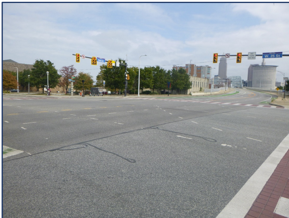
Photo 510-3 – West Station, Areas of Cracking in Wearing Surface
