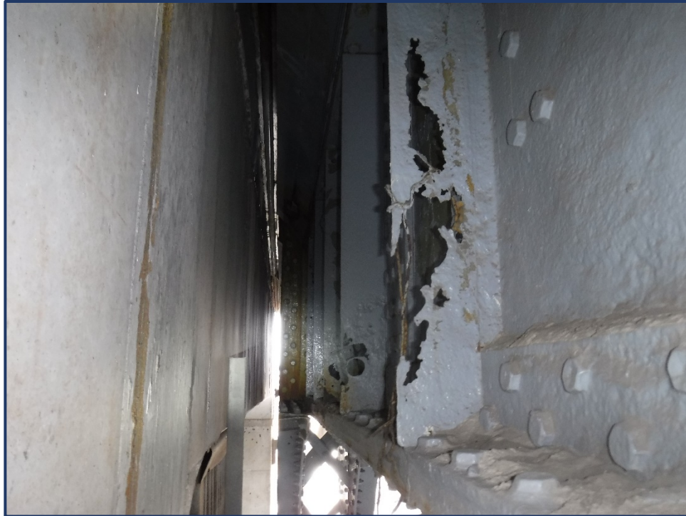
Photo 152-2 – Span 4, Upper FB0', Pitting of Floorbeam and Perforations in Stiffeners.
