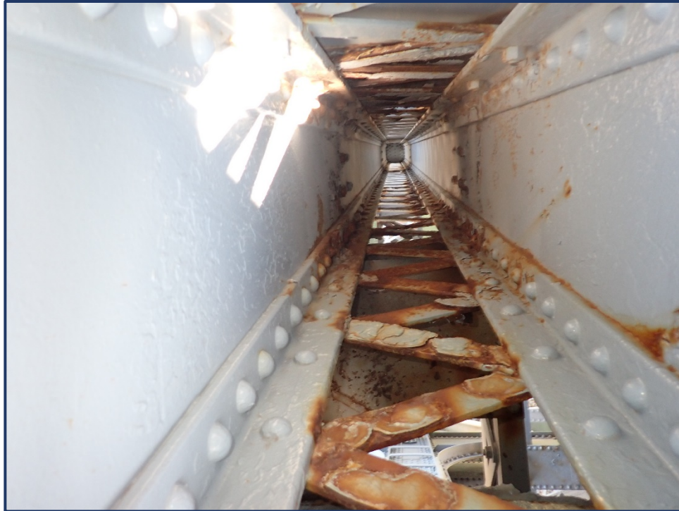
Photo 120-2 – Span 4, North Truss, U1'-L2', Active Corrosion extending down from Upper Deck
