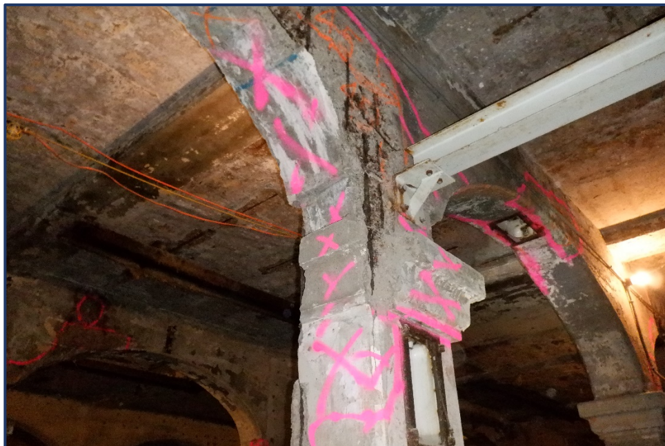
Photo 205-4 – West Station, Column Spalling with Exposed Reinforcing
