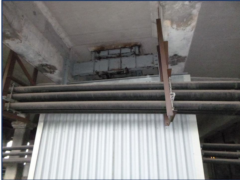
Photo UT-1 – Deteriorated Lower Deck Utility Junction Chamber Support.
