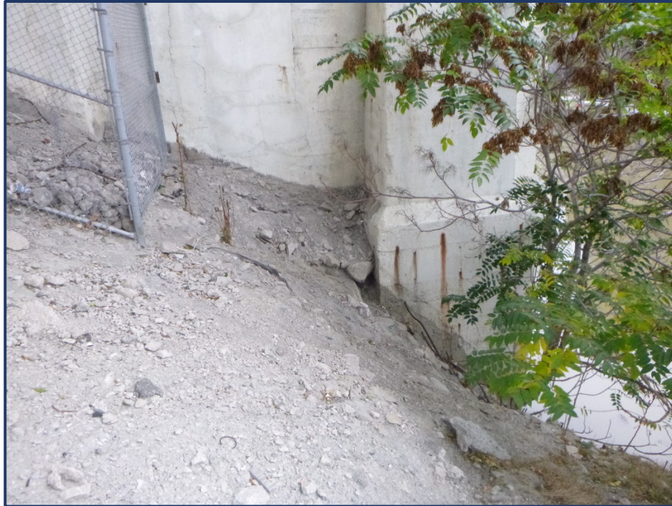
Photo APR-1 – Erosion of Embankment on West Side of Pier 3
