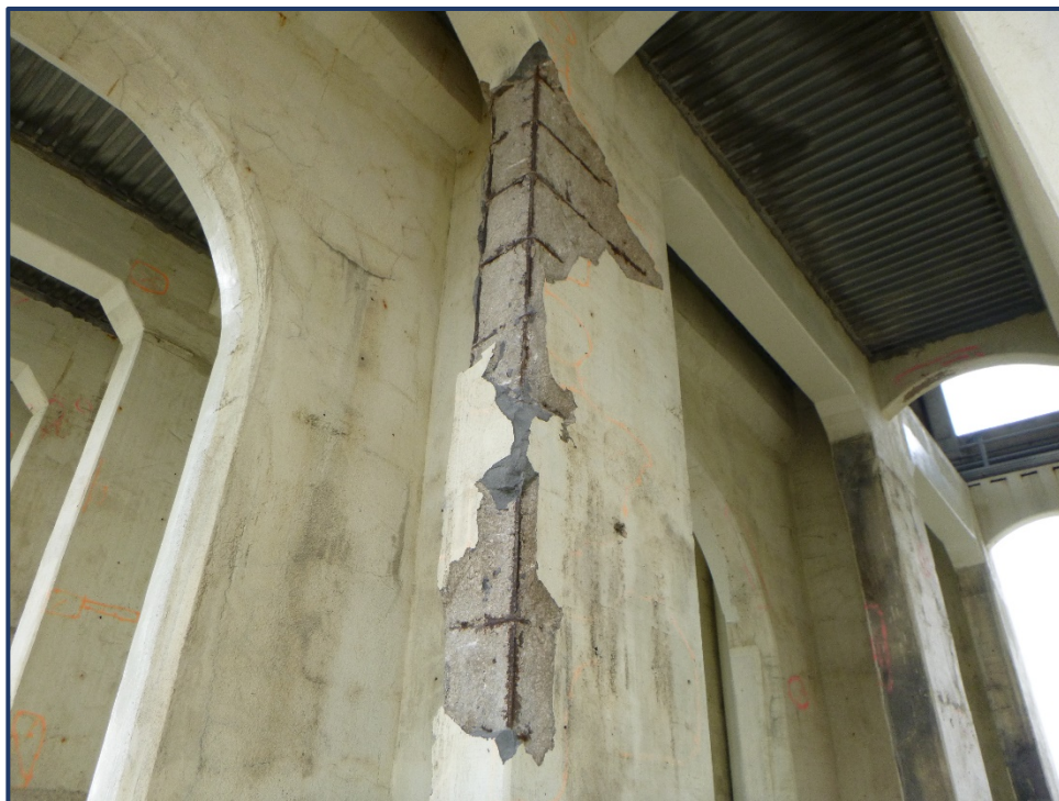
Photo 144-5 – Span 8, South Interior Arch, Spalling of Arch Column
