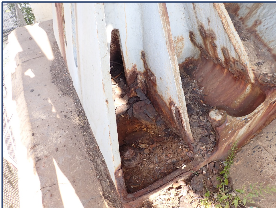
Photo 313-4 – Span 4, South Truss, L0' Bearing, Anchor Bolt & Nut Section Loss
