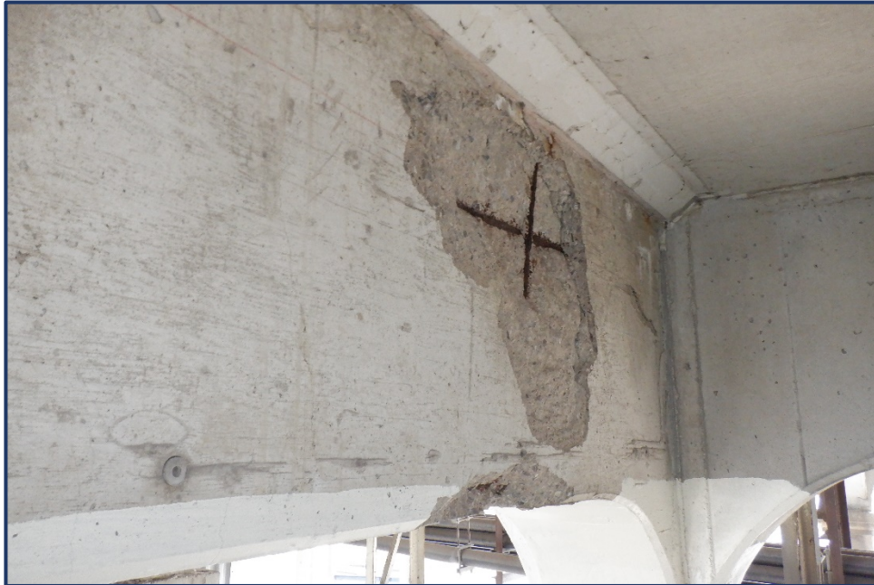
Photo 155-3 – Span 3, Upper Deck FB 3, Center Bay, Spalling and Delamination
