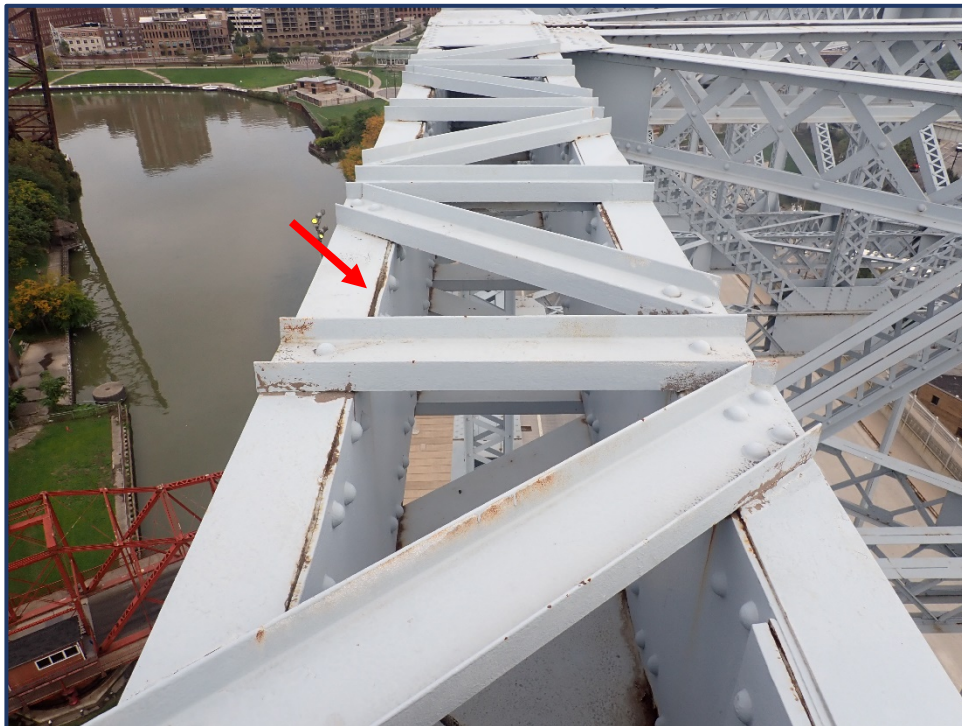
Photo 120-1 – Span 4, North Truss, U11-U12, Active Pack Rust between Web Plate and Flange Angles.
