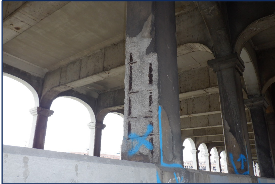
Photo 144-6 – Span 7, North Interior Arch, Spalling of Arch Column
