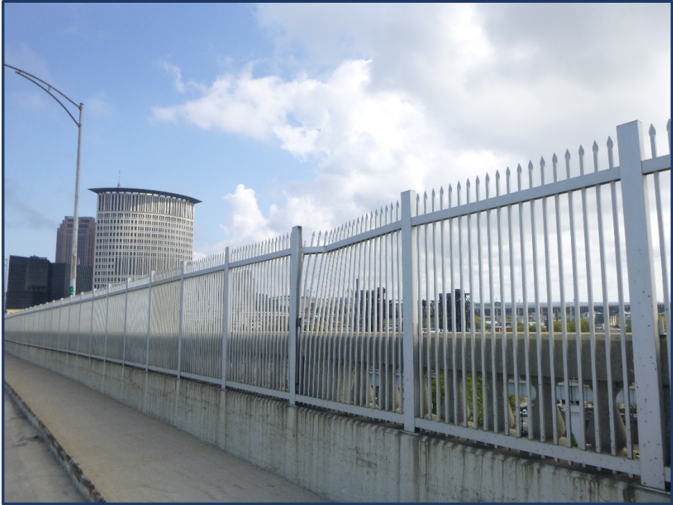
Photo 331-2 – South Rail Fence, Area of Damage in Span 5
