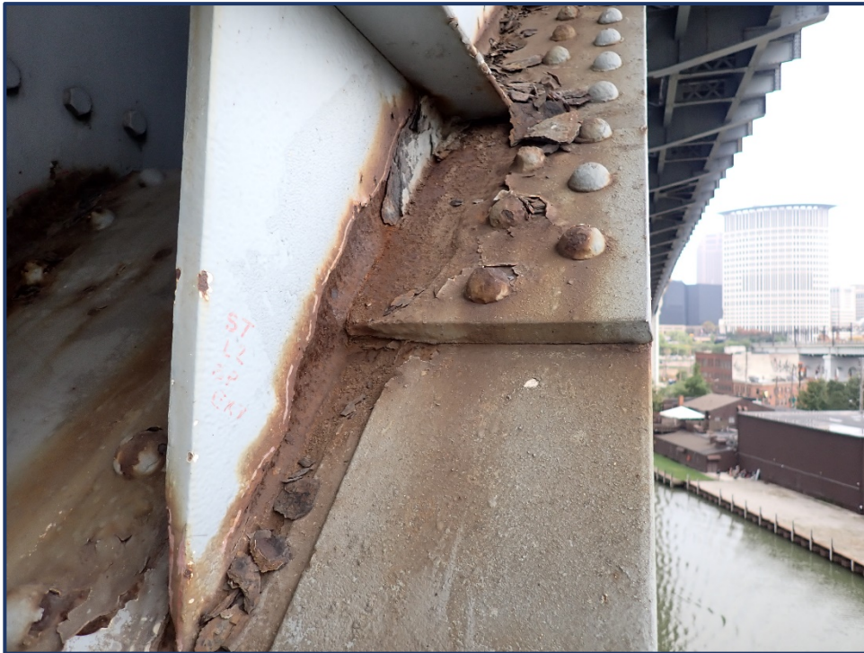
Photo 162-1 – Span 4, South Truss, L2 South Gusset Plate, Active Pitting along L1-L2
