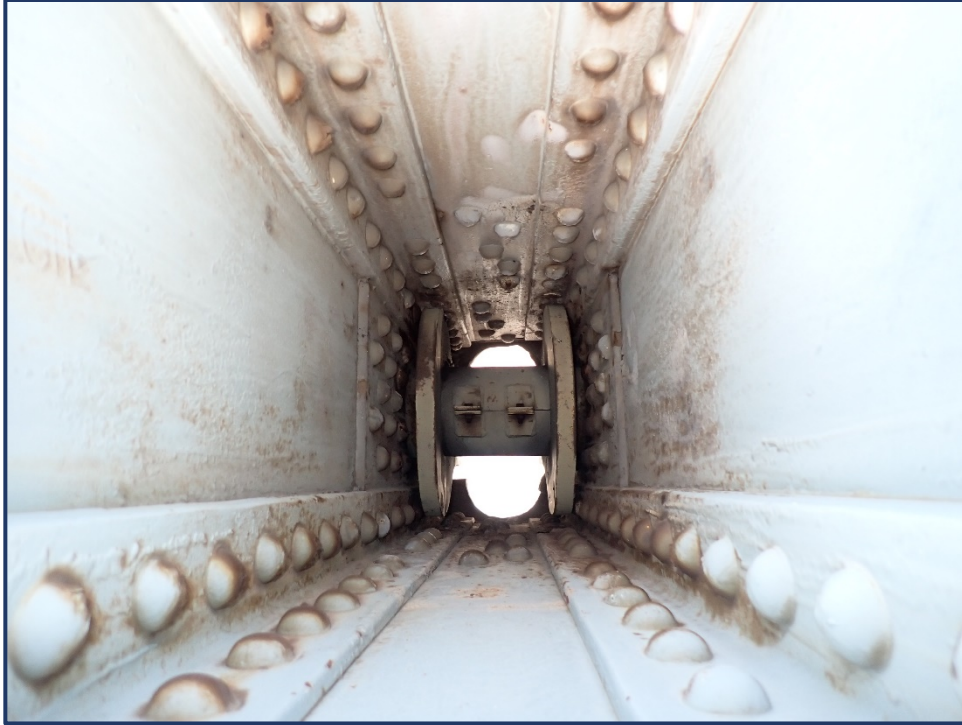
Photo 120-6 – Span 4, North Truss, L10, Reactivating Pitting around Hanger Pin
