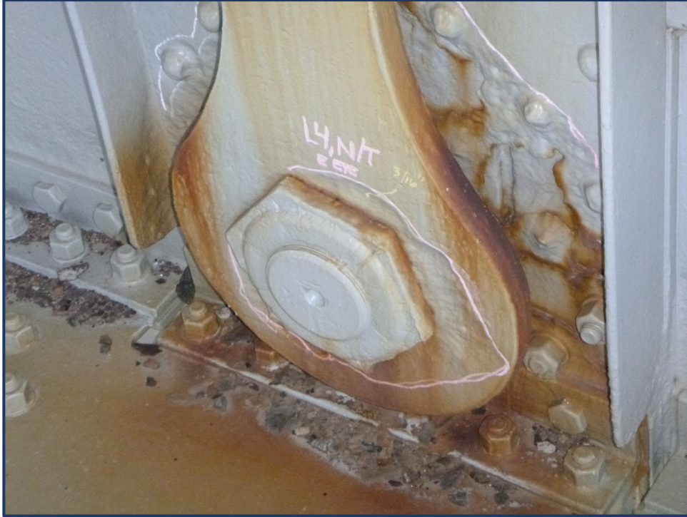
Photo 161-1 – Span 4, North Truss, Hanger Connection at Lower FB4, Pitting around Pin
