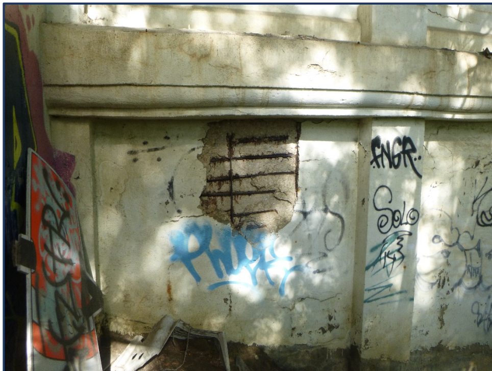
Photo WW-1 – Span 1A South Wingwall, Area of Spalling with Exposed Reinforcing
