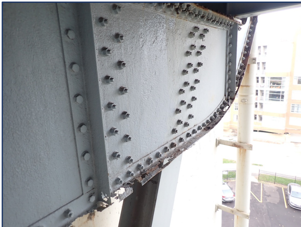
Photo 152-3 – Span 4, Lower FB0, North End, Perforations and Active Corrosion of Bottom Flanges
