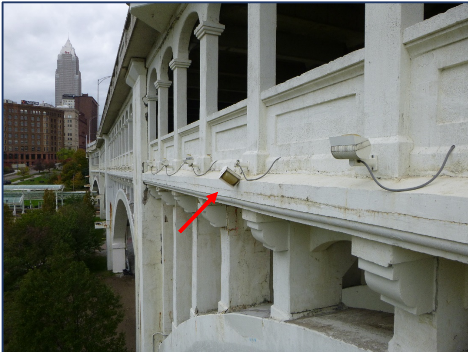
Photo UT-6 – Broken Architectural Light, Span 8 North Fascia
