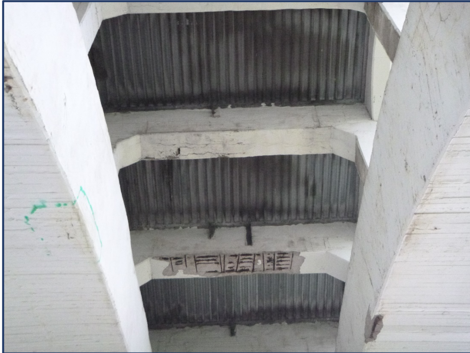
Photo 155-1 – Span 3, Lower Deck FBs, South Bay, Cracking, Delamination and Spalling with Exposed Reinforcing
