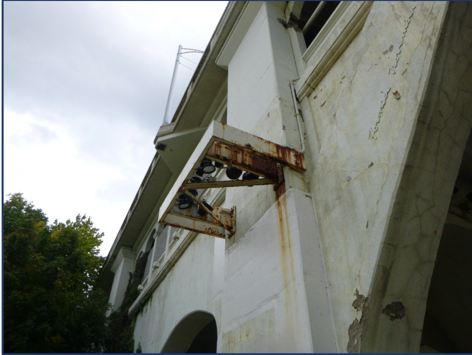
Photo UT-5 – Typical Corrosion and Minor Section Loss on Tower Light Brackets
