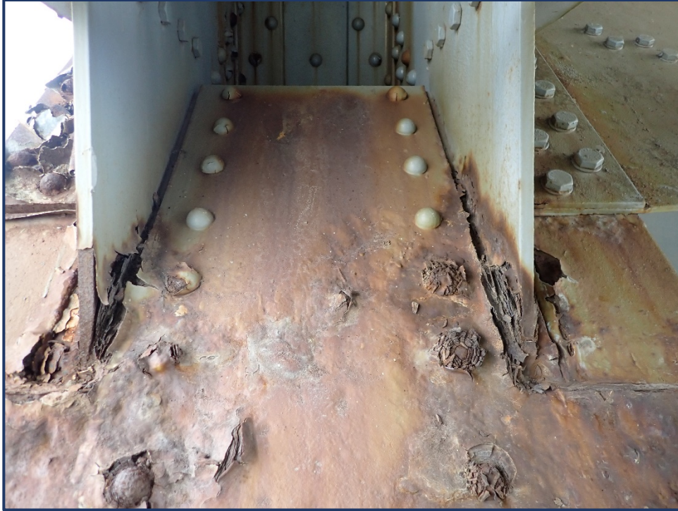
Photo 162-2 – Span 4, South Truss, L2' Gusset Plates, Active Pitting & Pack Rust
