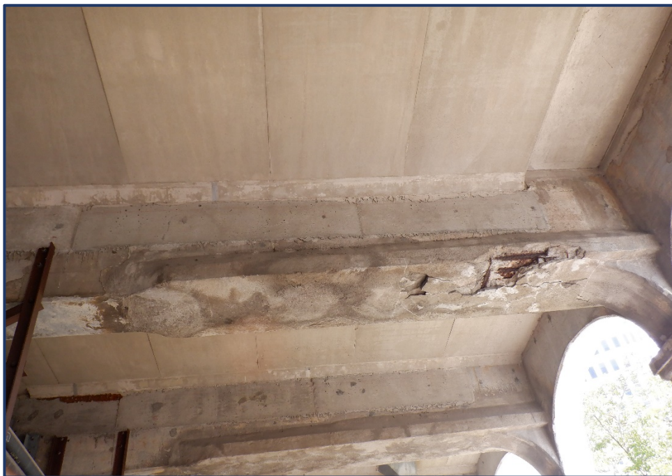
Photo 155-3 – Span 13, Upper Deck FB 6, South Bay, Spalling and Delamination
