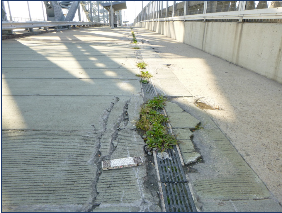
Photo CS-2 – Span 4 North Sidewalk, Delamination and Cracking along Longitudinal Drain
