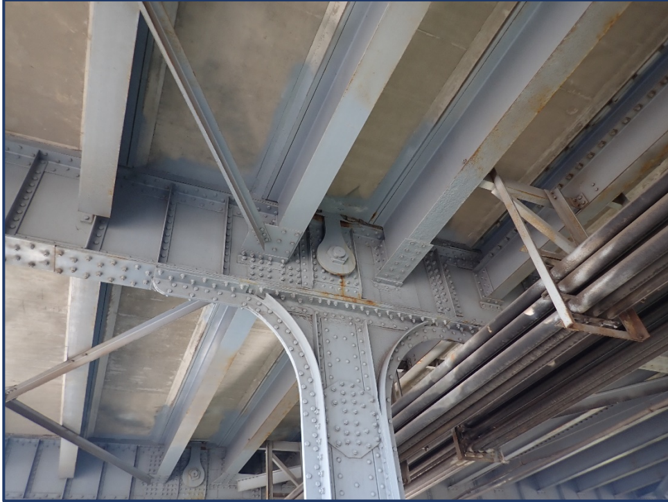
Photo 113-1 – Span 4, Upper Deck Stringers, Typical Surface Corrosion and Minor Pitting on Stringer Ends
