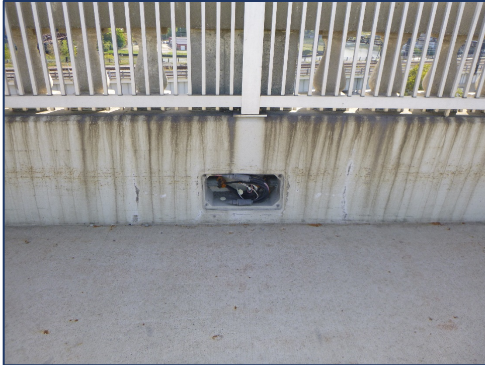
Photo UT-3 – Missing Electric Junction Box Cover, South Railing, Span 7
