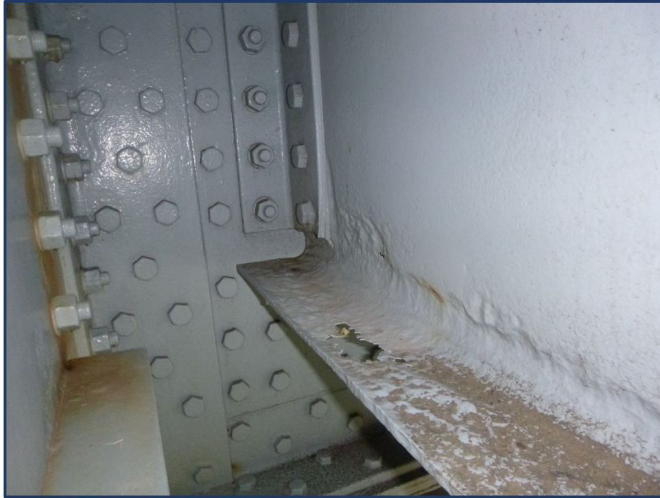
Photo 113-3 – Span 4, Upper Deck Stinger E, Bay 2-3, 5" L x 2" W Perforation at FB3
