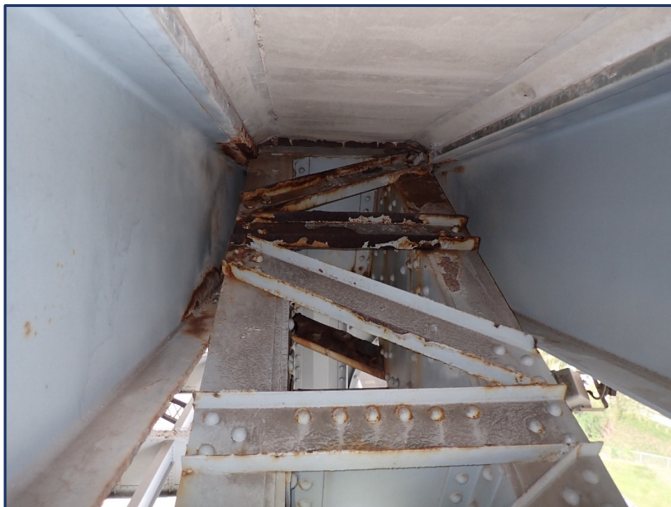
Photo 515-1 – Span 4, Peeling Paint and Surface Corrosion Below Upper Deck
