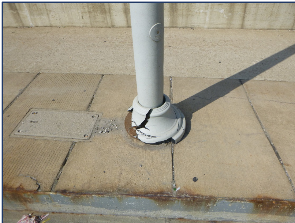
Photo UT-4 – Broken Light Pole Base Cover on North Sidewalk
