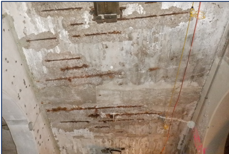
Photo 12-2 – West Station, Typical Scattered Deck Spalling with Saturation and Efflorescence
