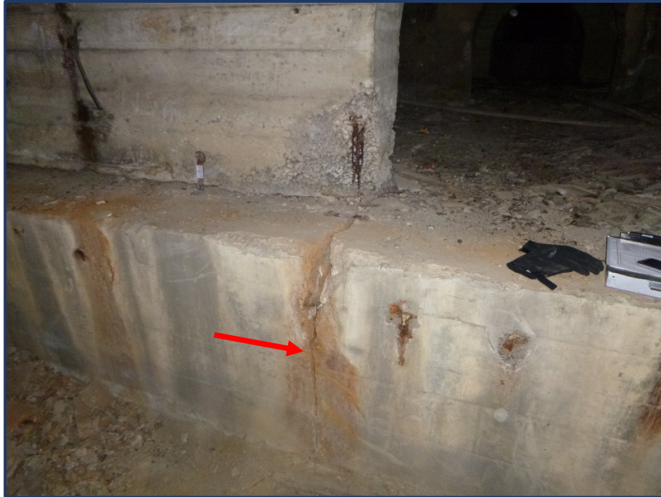
Photo WW-2 – West Abutment Chamber, Crack Through Footing at Tower B
