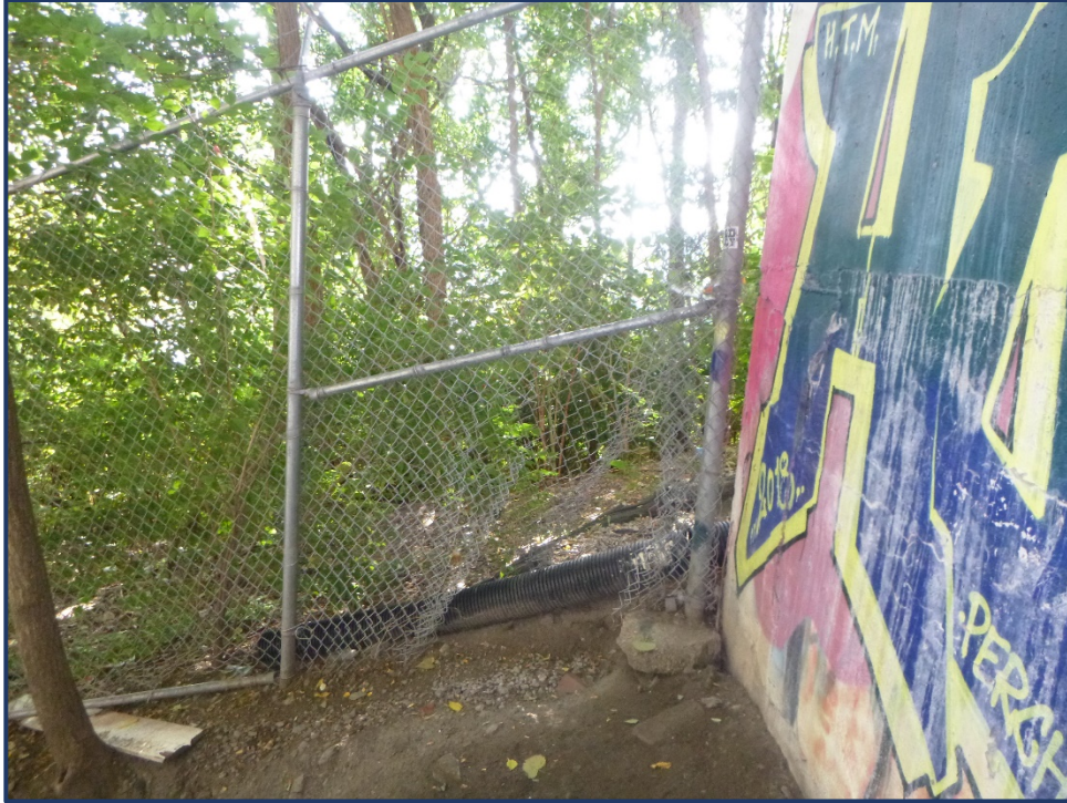
Photo APR-5 – Hole Cut in Vandal Fence Fabric at South Corner of Span 1A
