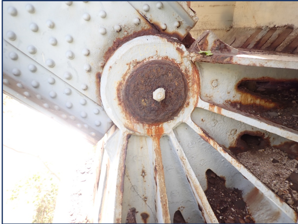
Photo 313-3 – Span 4, North Truss, L0 Bearing, Missing Pin Cover Plate
