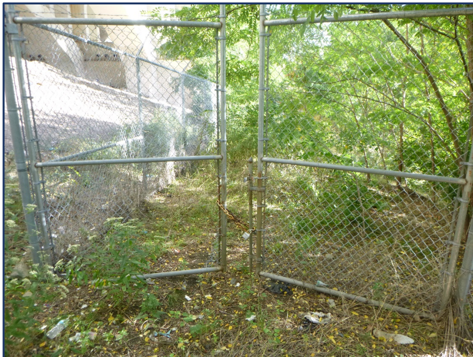
Photo APR-4 – Hole Cut in Vandal Fence Fabric at South Corner of West Abutment
