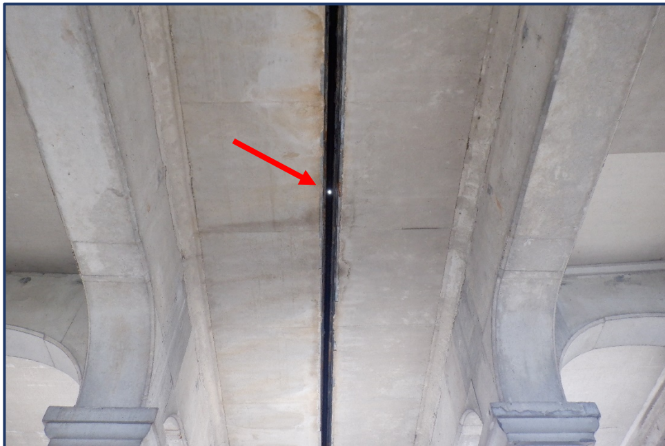
Photo 300-3 – Pier 10 Joint, 4' Section of Seal Tearing
