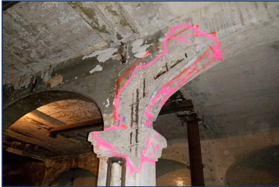
Photo 110-1 – West Station, Spalling of Concrete Beam
