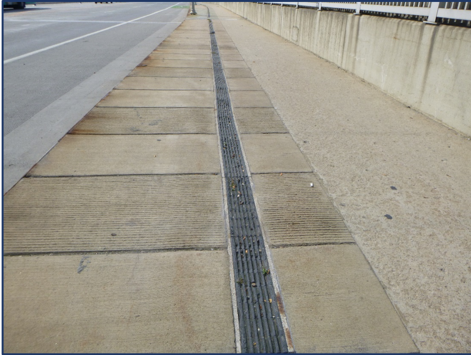
Photo 815-3 – North Sidewalk Longitudinal Drain, Typical Clogging with Debris
