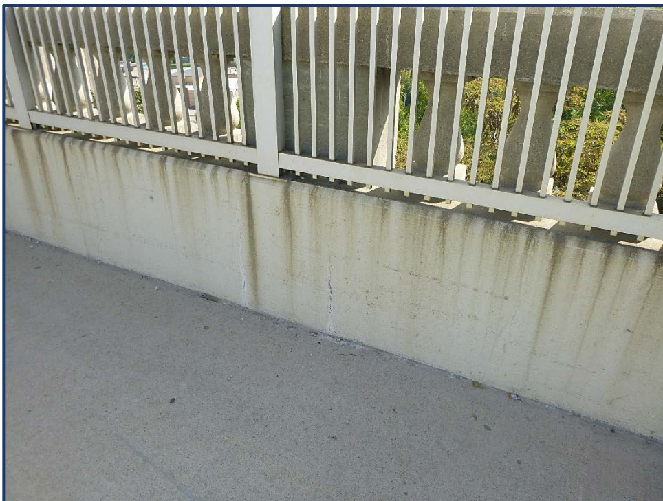
Photo 331-1 – South Rail, Typical Cracking and Staining
