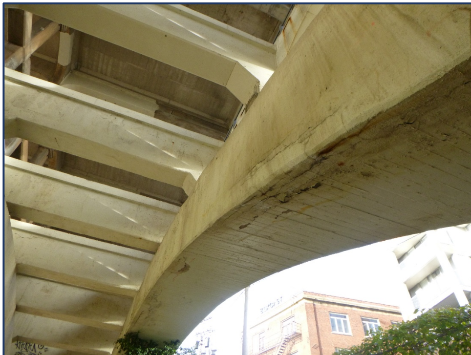
Photo 144-3 – Span 1, North Exterior Arch, Map Cracking and Delamination of Arch Rib
