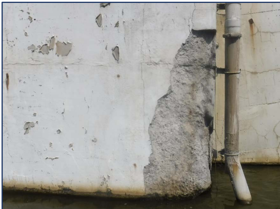
Photo 210-2 – Pier 3, Southeast Corner, Spalling at Waterline
