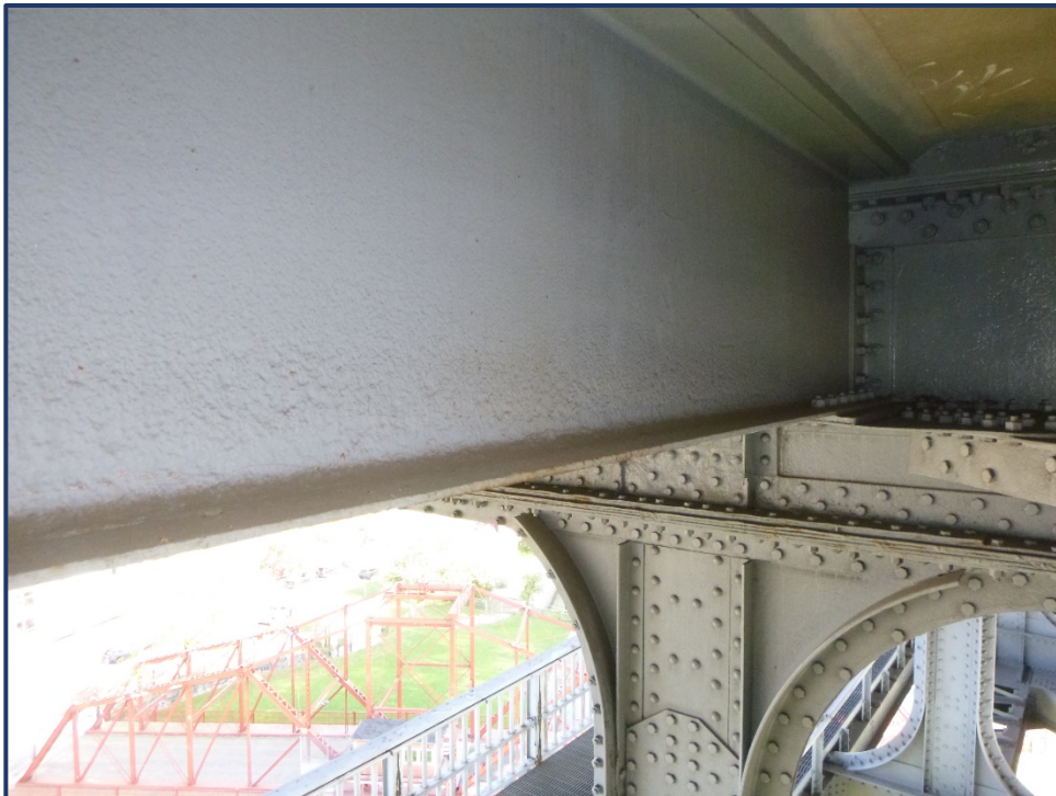
Photo 113-2 – Span 4, Upper Deck Stinger E, Bay 4'-5', Active Pitting Corrosion and Painted over Pitting
