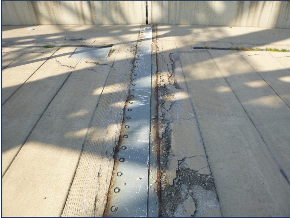
Photo 300-2 – Joint in Span 4 at PP5, Spalling and Cracking of Header at North Sidewalk Expansion Joint
