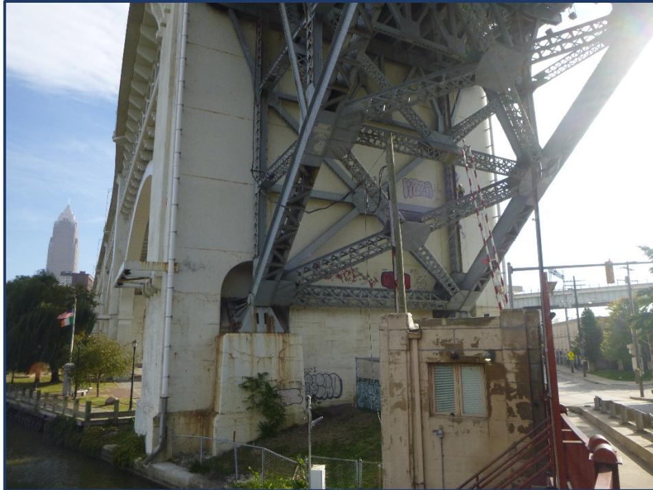
Photo 210-1 – Pier 4, West Face, Typical Map Cracking in Lower Portion
