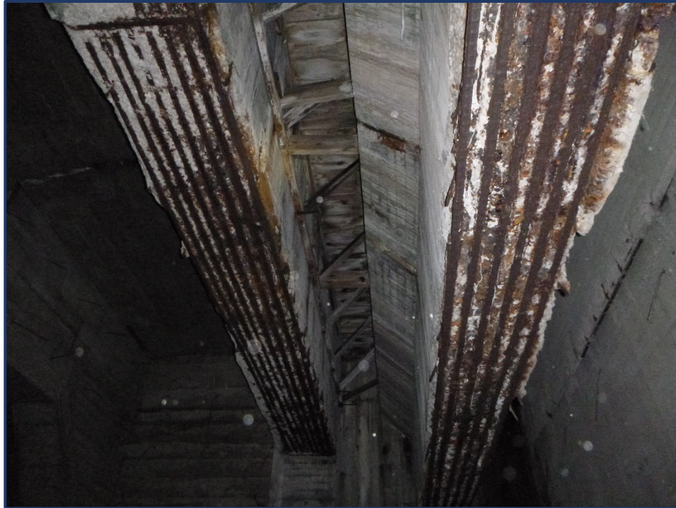
Photo 155-4 – East Abutment Chamber Floorbeams, Typical Spalling
