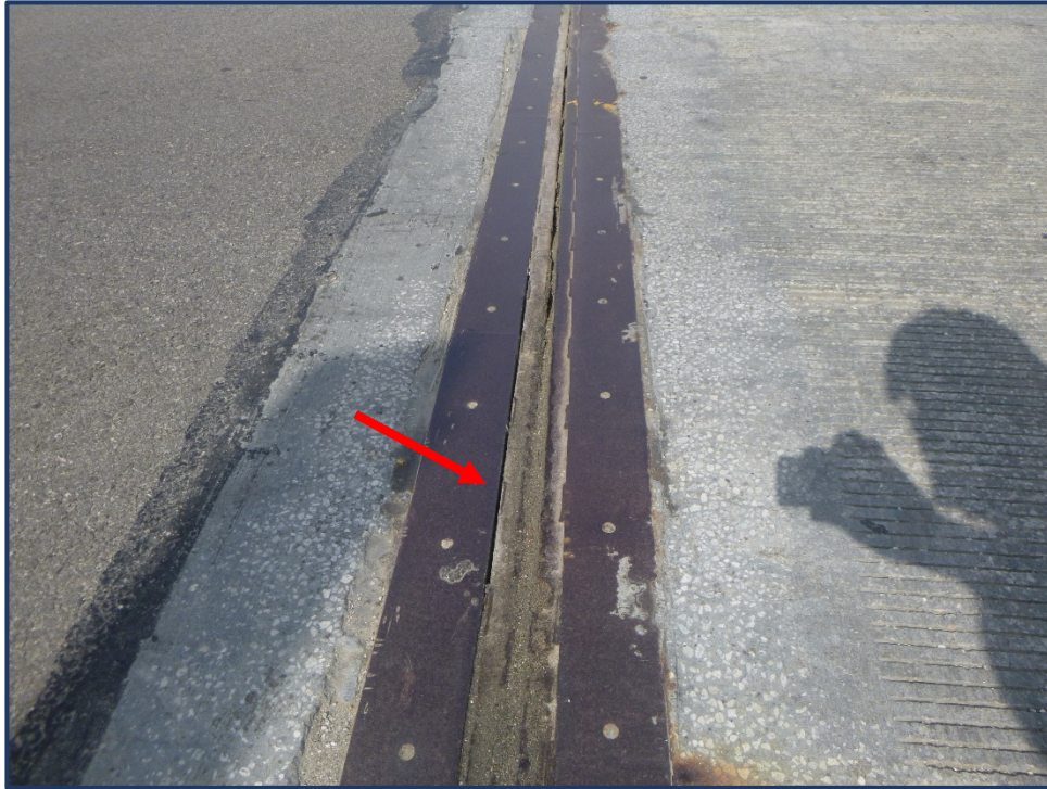
Photo 300-4 Joint 1A, 2' Section of Broken Intermittent Fillet Welds in Joint Armor
