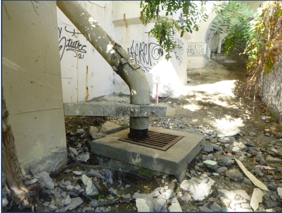
Photo 815-1 – Pier 1, East Face, South Downspout Fully Clogged.
