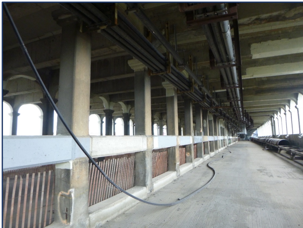
Photo UT-2 – Sagging Utility Line on Maintenance Deck
