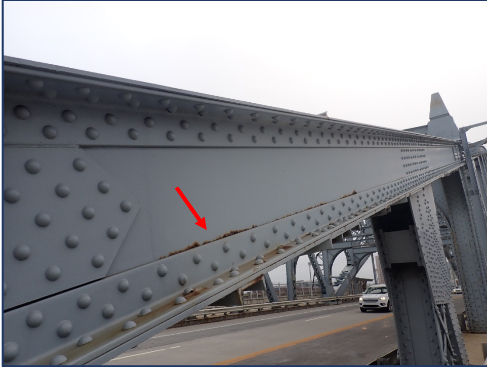
Photo 120-1 – Span 4, South Truss, U0-U1, Active Pack Rust between Web Plate and Flange Angles.
