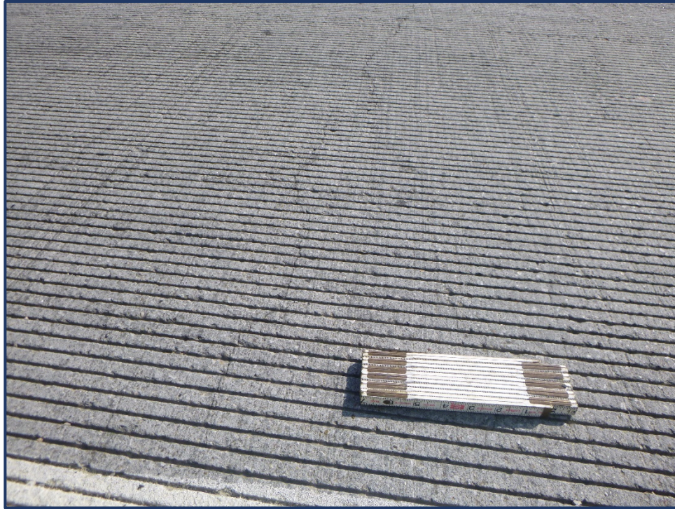
Photo 510-2 – Map Cracking in Wearing Surface
