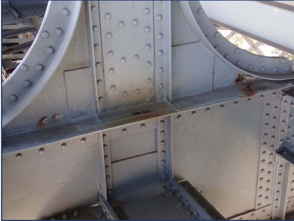
Photo 152-4 – Span 4, Lower FB9 at South Truss, Pitting and Perforations
