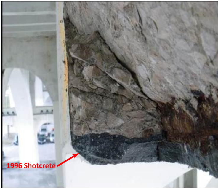
Photo 5 – Spalled Original Concrete & Secure 1996 Shotcrete Patch, Span 7 South Interior Arch Rib.
