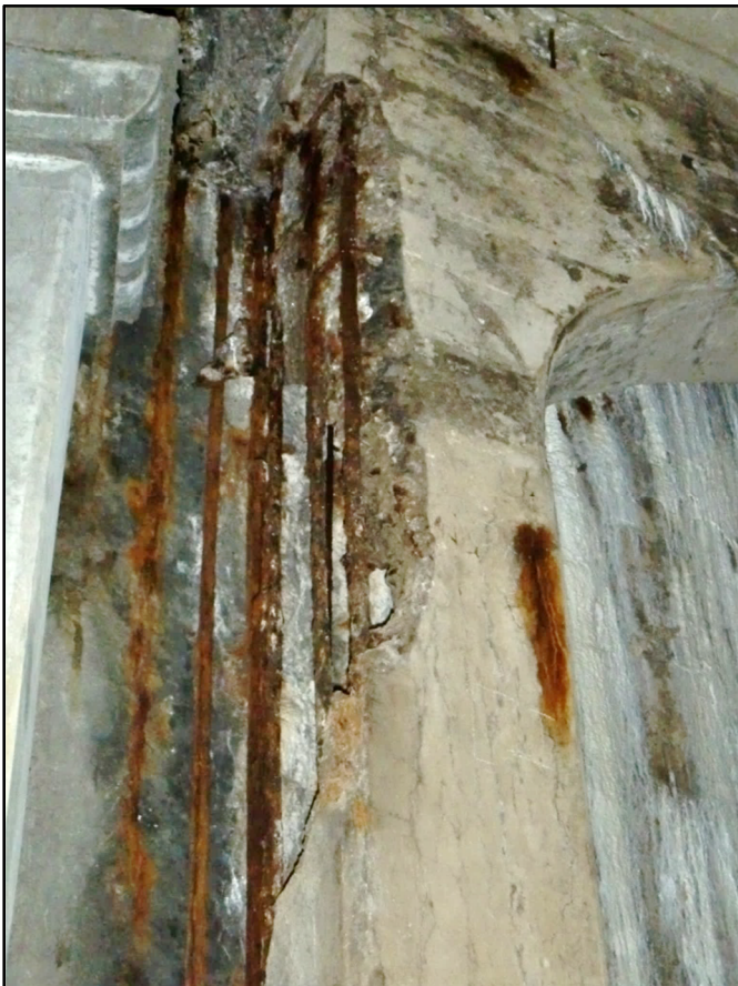
Photo 8 – 60% Section Loss, Column M22, East Station.
