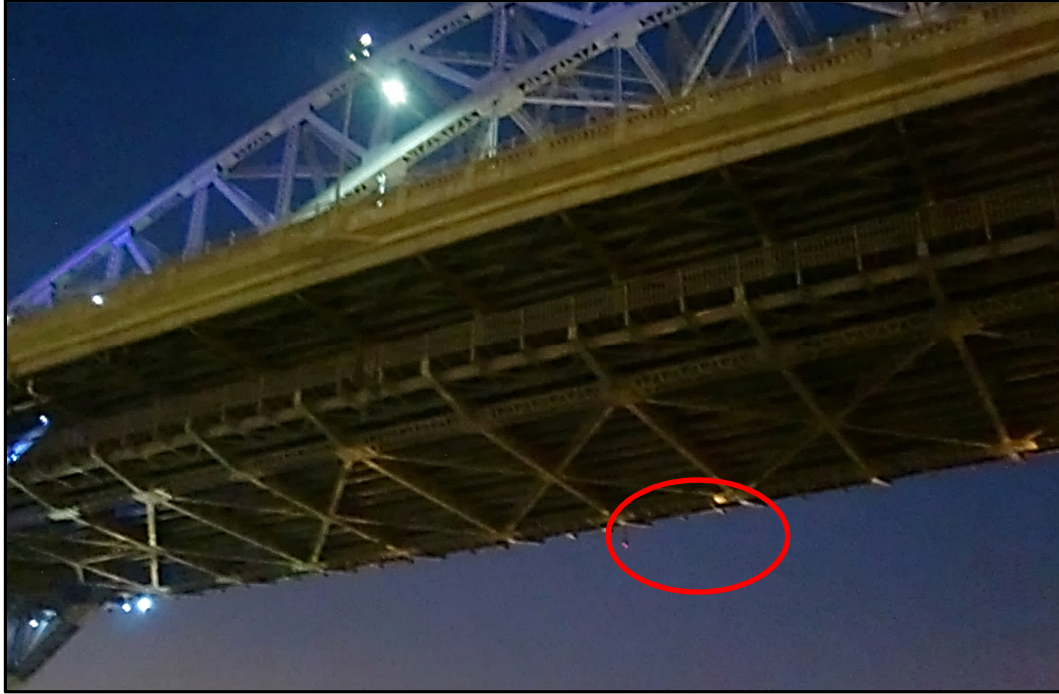
Photo 12 – Typical Ineffective Illumination of Navigation Light (East Edge of Channel, South Face circled).
