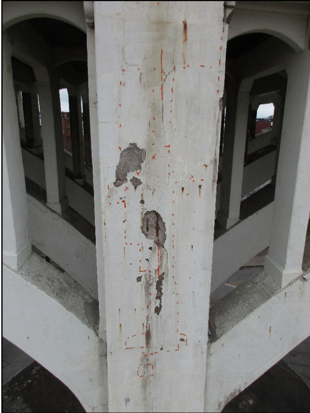
Photo 7 – Deep Concrete Deterioration, Pier 6 South Lower Deck Pier Shaft.
