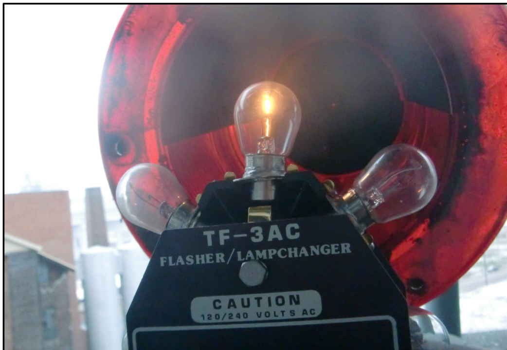
Photo 11 - Power Verification of Navigation Light (West Edge of Channel, South Face shown).
