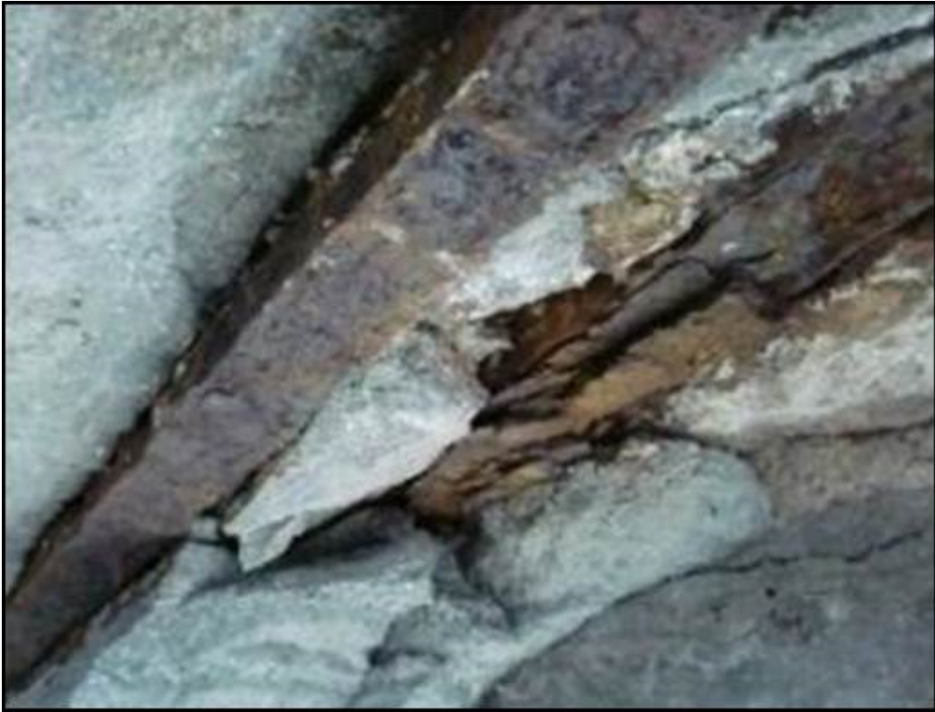
Photo 4 – Reinforcing Steel with Active Corrosion, Lower Deck Floorbeam 14, South Bay, Span 6.
