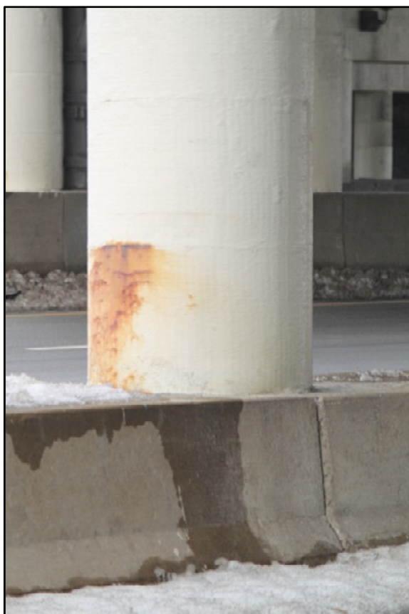
Photo 10 – Active Concrete Corrosion Beneath FRP Wrap, Pier 1, CUY-71-1679 (Fulton Road over I-71).
