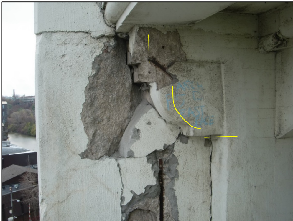
Photo 6 – Spalled & Loose Concrete Due to Ineffective Bond Breaker (Location denoted in yellow), Pier 5 Lower Deck Pier Shaft & South Lower Deck Corbel 1, Span 6.
