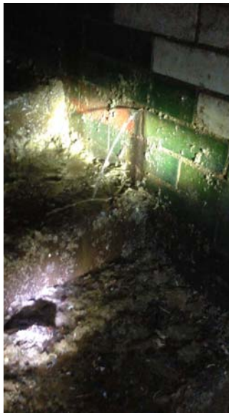
Figure 12: Water Penetrating through Walls
