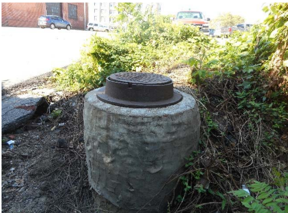
Figure 14: Partially Plugged Manhole as shown in Figure 11
