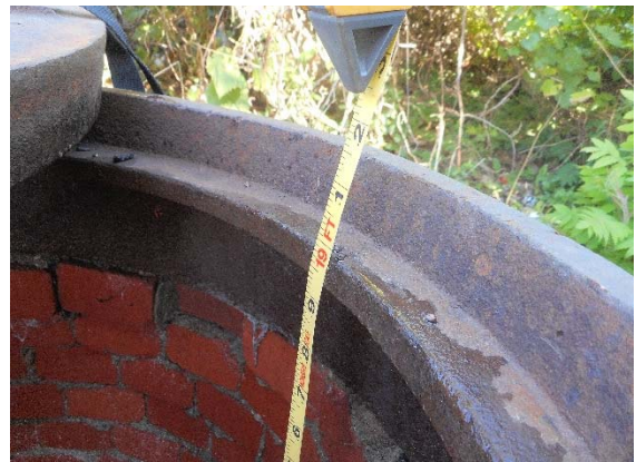
Figure 15: Water Depth in Partially Plugged Manhole
