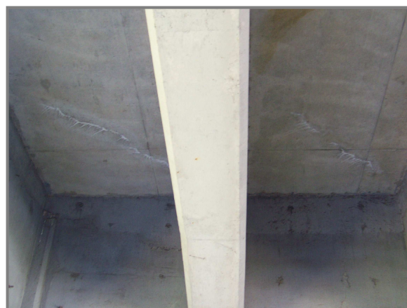
Photo 2 – Minor diagonal cracking in Bays 2 and 3 at the extreme east end of Section P.
