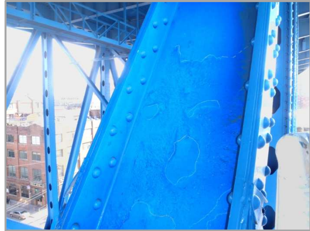
Photo 9– Member U52-L53 of the north truss with heavy web section loss.
