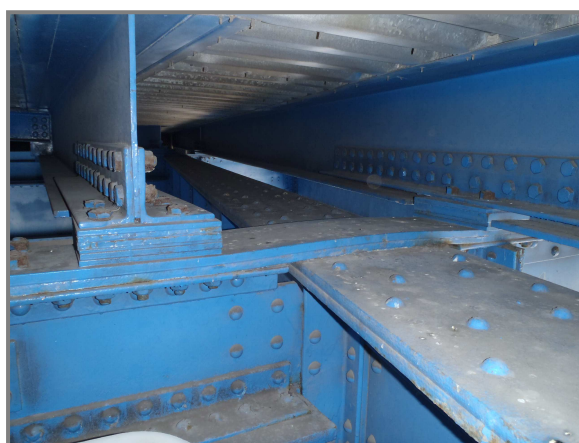
Photo 7 – Typical framing in Section N, stringers supported floorbeams that are framed into girders.
