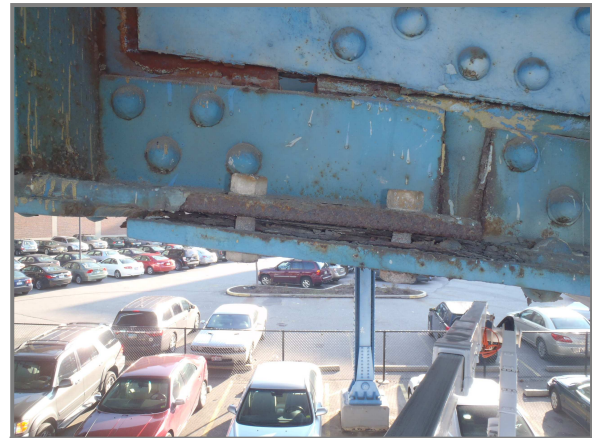
Photo 14 – Pack rust between South Girder bottom flange and wind shear plate at Bent 29. Note bolts have backed off nuts.
