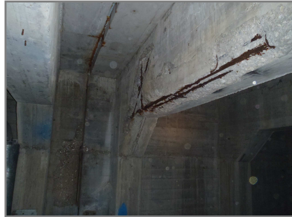
Photo 3 – The west face of Bent 21 in Section D of the west approach exhibits a large spalled area with exposed reinforcement.
