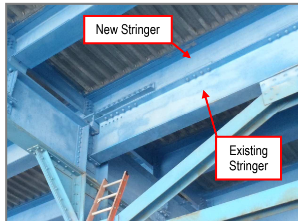
Photo 11 – Forward Section showing t-shaped stringer added in rehabilitation on top of existing stringer.
