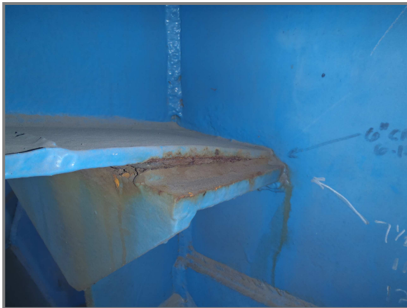
Photo 6 – Cracked weld between the seat and south bracket at Column K2 in Section K.
