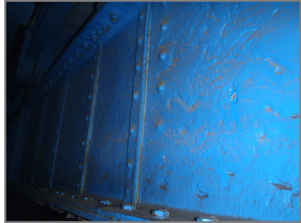
Photo 13 – Typical pitting of the east face of Floorbeam 14 at mid-beam. Note the removal of vertical stiffener legs in this area.
