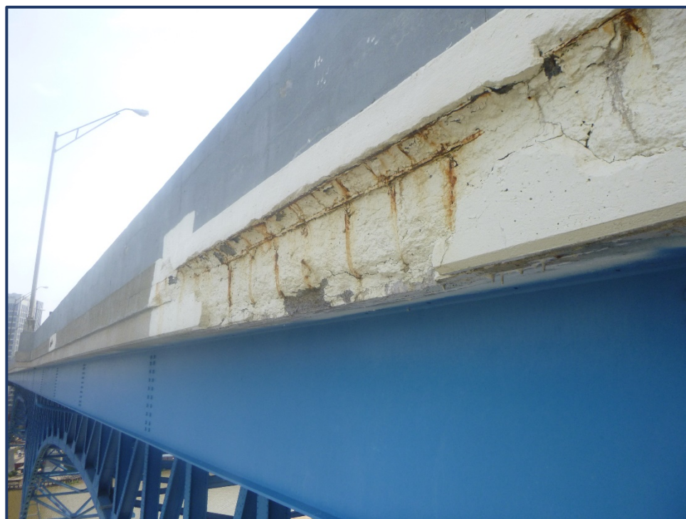
Photo 12-2 – Deck Edge Spalling and Delamination in Unit II
