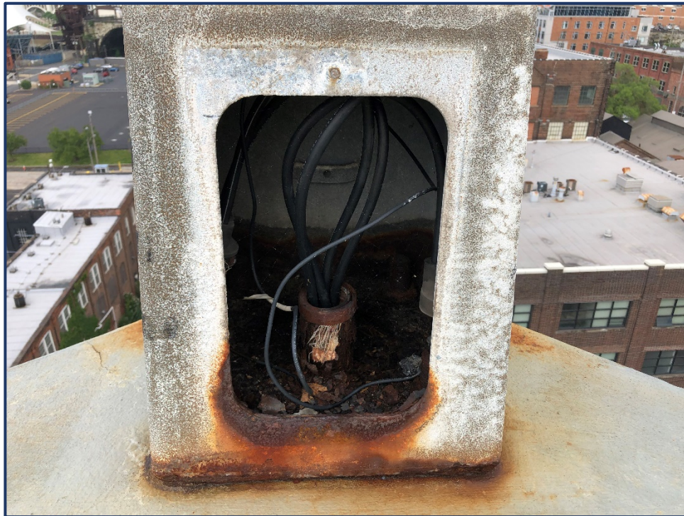
Photo LI-1 – Typical missing utility cover at light pole, Span 5 over Elm Street
