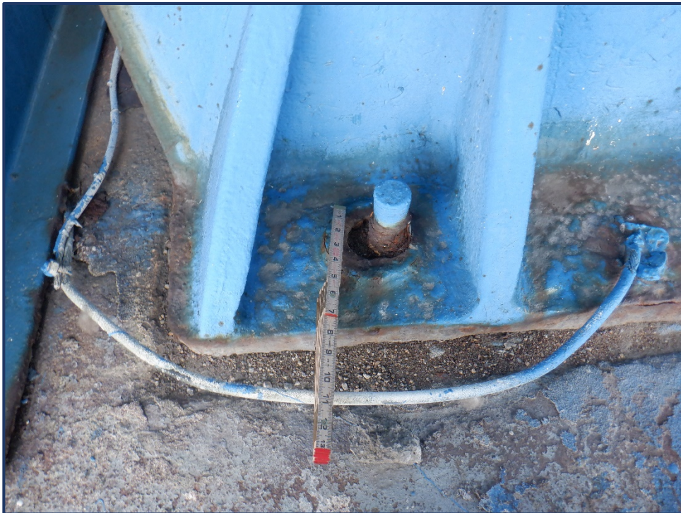
Photo 311-1 – Unit II, Pier 0, South Truss Bearing, Section Loss of Bearing and Anchor Bolt Nuts
