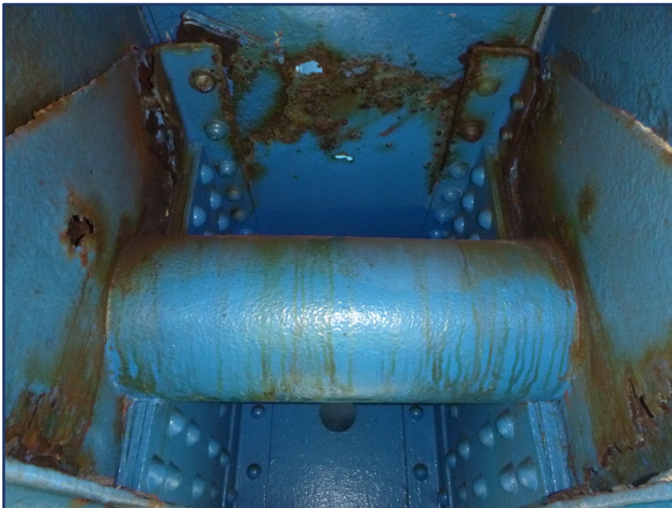
Photo 161-1 – Unit II, Span 9, North Truss, Painted over Pitting on Pin with Rust Staining
