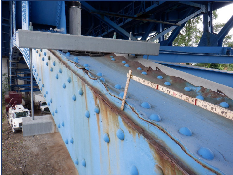
Photo 120-7 – Span 1, South Truss, L8-L9, Distortion of Top Flange Plate due to Pack Rust
