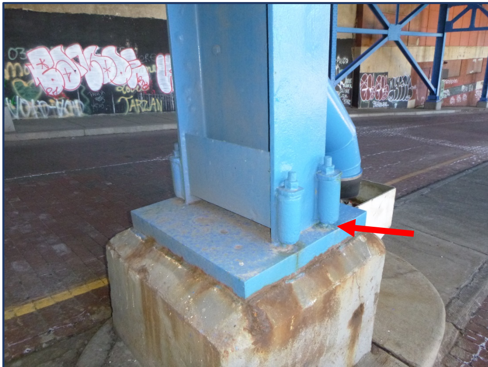
Photo 202-1 – Unit III, Bent 8 Center Column, Painted Over Section Pitting and 75% Loss of Anchor Bolts
