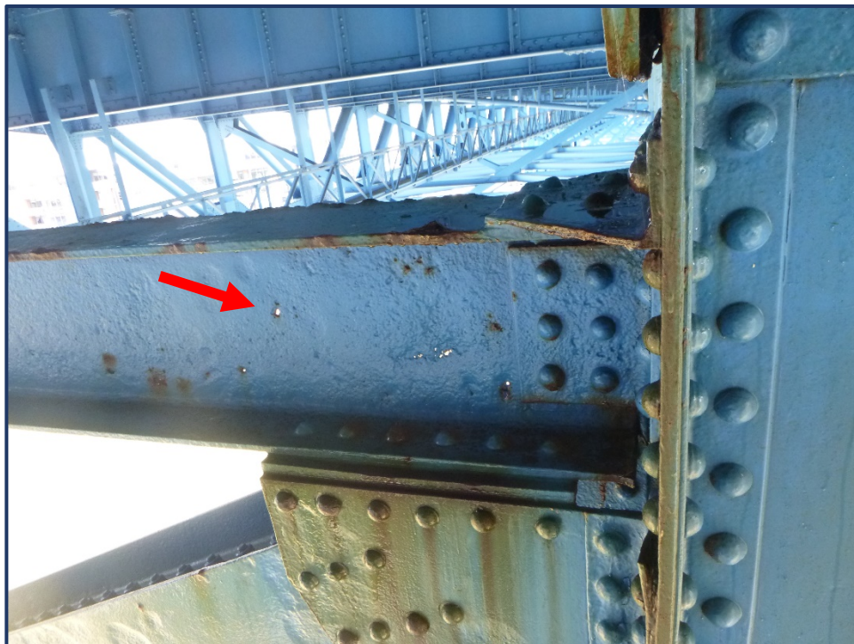
Photo 120-8 – Typical Painted over Section Loss with Perforations in Sway Bracing
