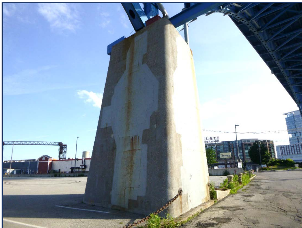
Photo 205-2 –Unit II, Pier 7 North, Patching and Rust Staining
