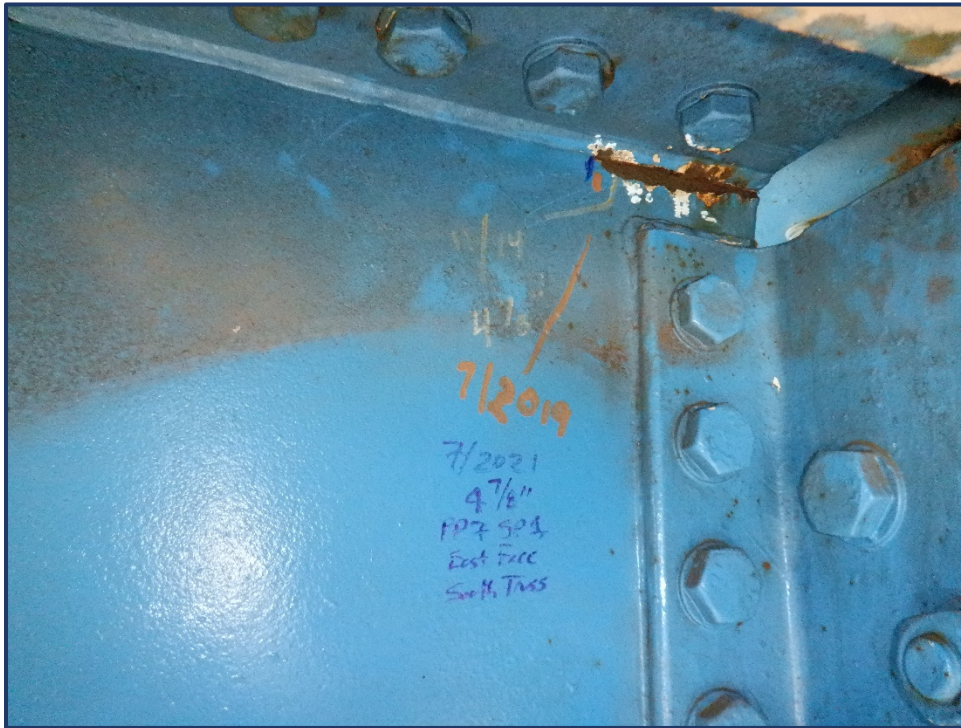
Photo 152-5 – Unit II, Span 1, FB 7 at South Truss, Crack in Top Flange Cope Exhibiting Slow Growth
