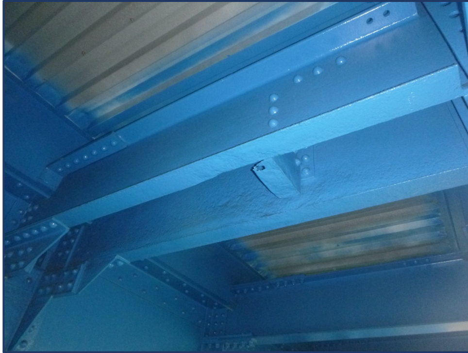
Photo 152-1 – Unit V, Painted of Section Loss of Floorbeam Cantilever at Abandoned Drainage Downspout Location
