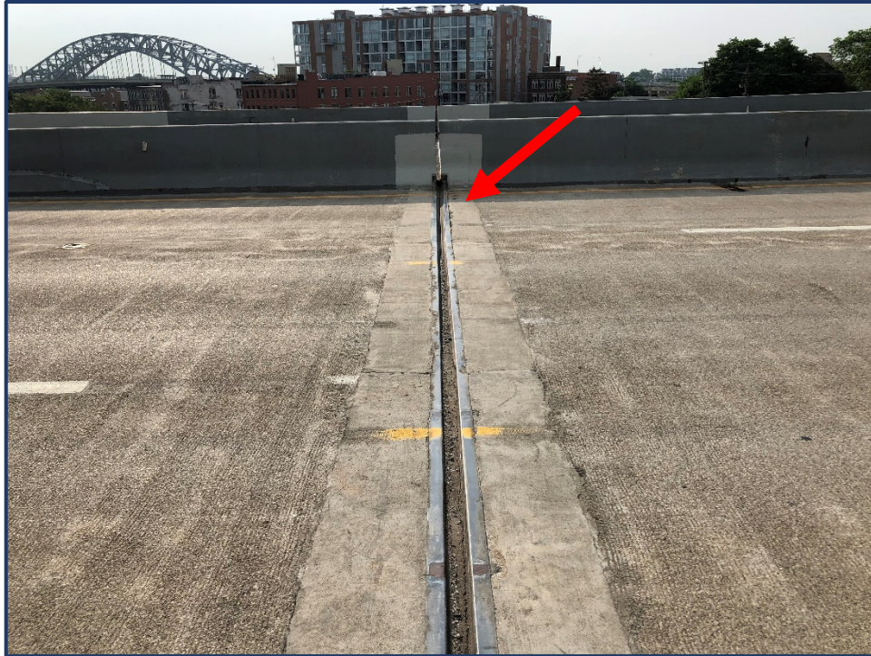
Photo 300-1 – Joint O Loose Joint Armor and Spalled Header
