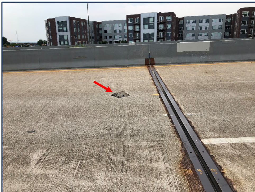
Photo 510-1 – Scattered Shell Spalling with Asphalt Patching in Wearing Surface
