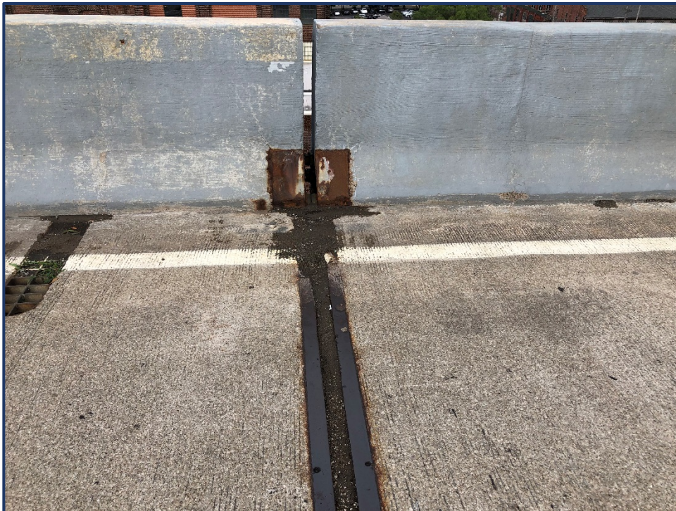
Photo 300-2 – Unit II, Span 4/5 Joint L1, Typical Rusting and Debris Impaction in Joint
