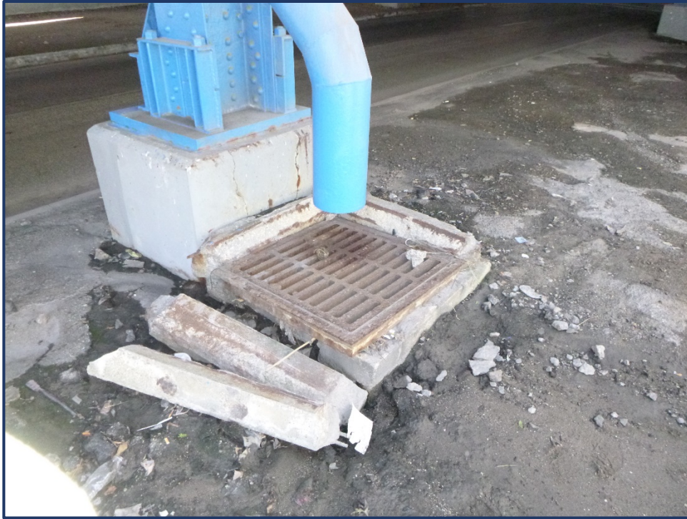
Photo 815-2 – Unit IV, Bent 15 Catch Basin, Heavy Spalling of Frame and Shifting Grate
