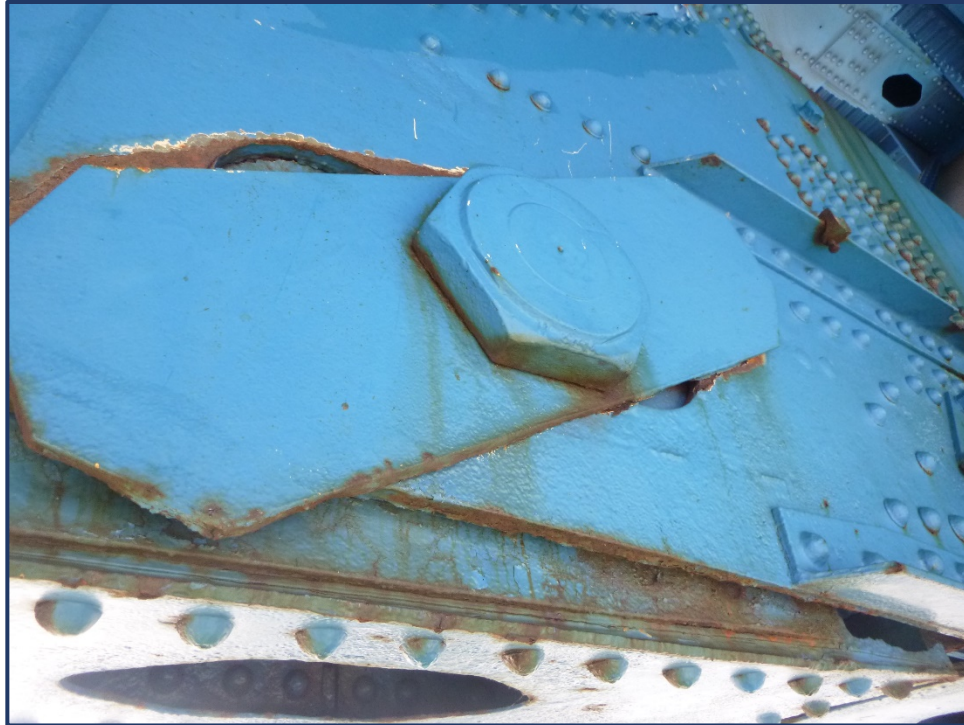
Photo 161-2 – Unit II, Span 9, South Truss, Rotated Pin Plate at L0
