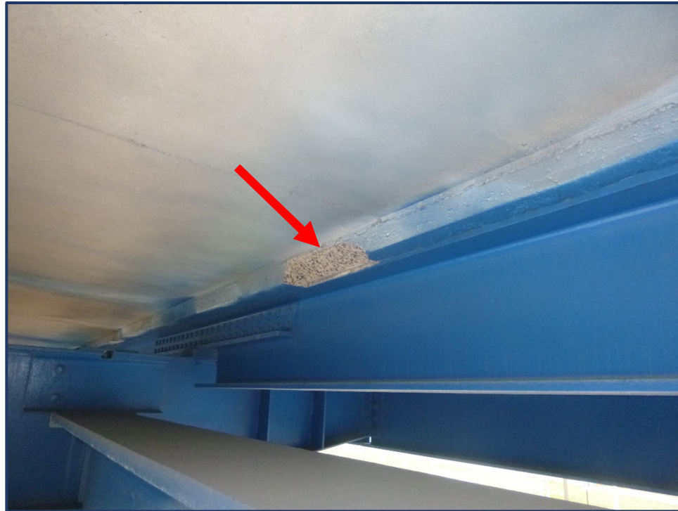
Photo 12-1 – Scattered Haunch Spalling in Unit I
