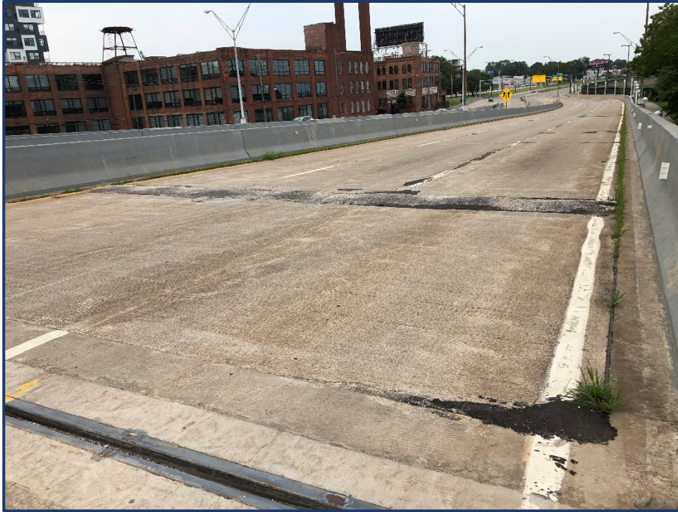
Photo 321-1 – West Approach Slab, Westbound, Areas of Patching and Heaving of Asphalt Joint
