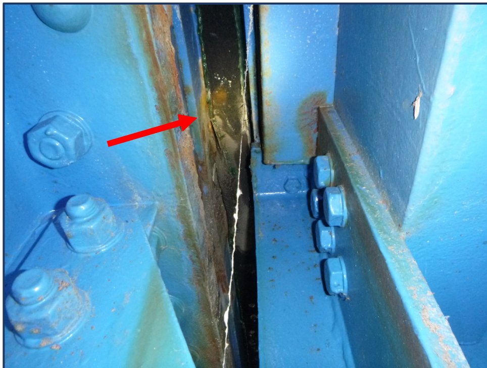
Photo 302-2 – Unit IV, Joint B4, Section of Compression Joint Seal Dislodged from Retainer, Eastbound Lane 1
