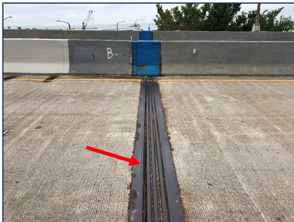
Photo 303-2 – Unit V, Joint B, Areas of Minor Seal Tearing
