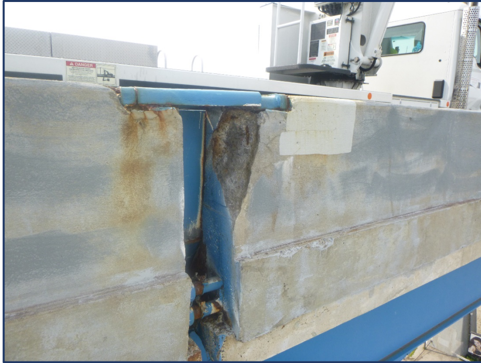
Photo 331-1 – Area of Parapet Spalling at Deck Joint.
