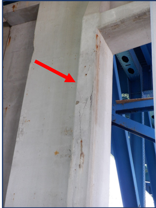
Photo 205-1 – Unit I, Unit P, East Pier, Delamination of North Column
