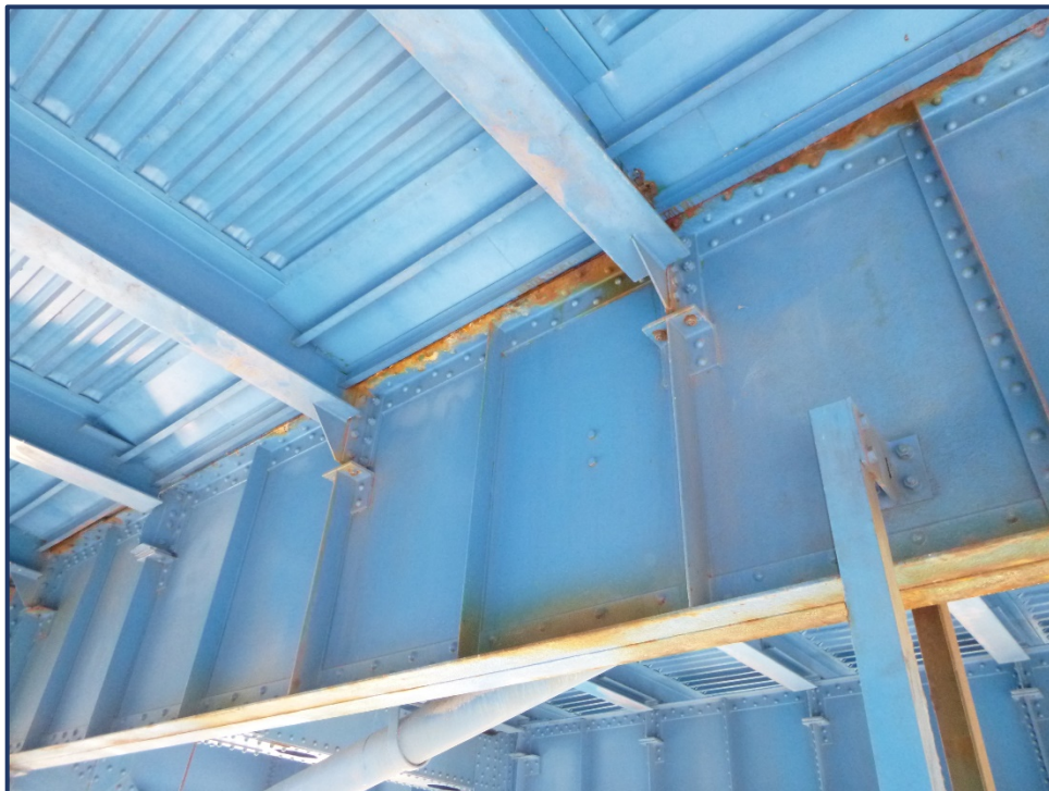
Photo 152-2 – Unit II, Span 2, FB 16, Active Surface Corrosion due to Deck Drainage
