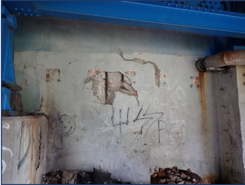
Photo 210-1 – Pier 37, East Face, Delamination and Spalling of Pier Wall
