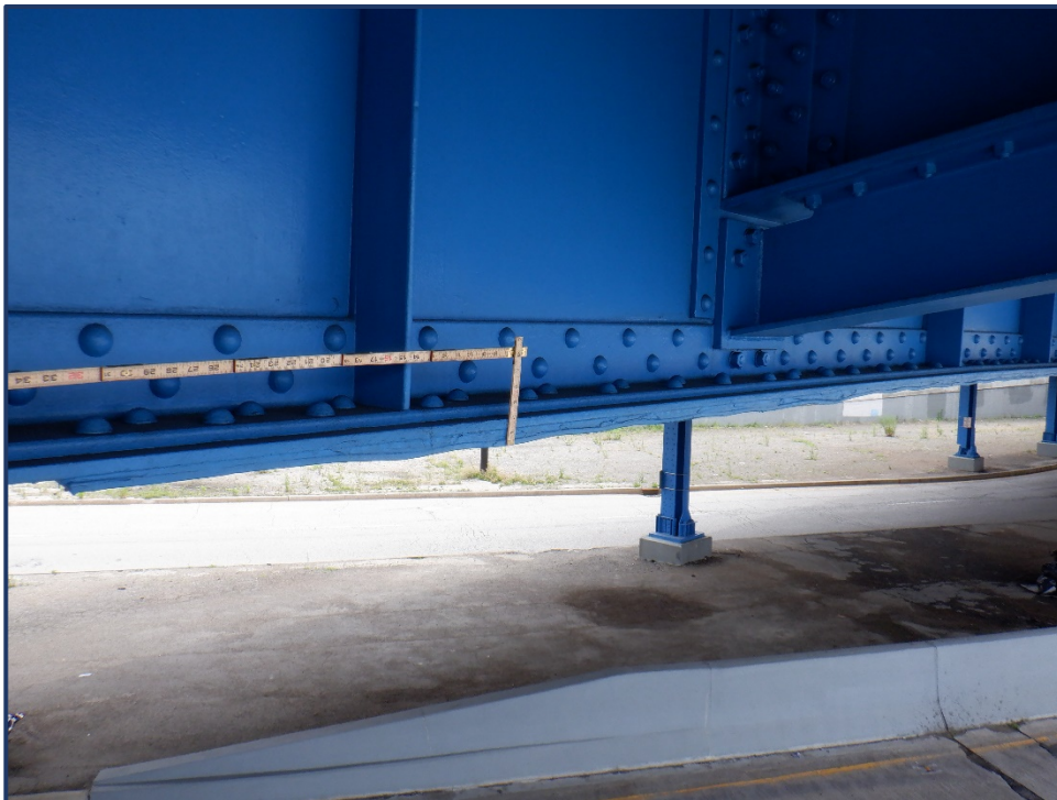
Photo 107-2 – Unit IV Girders, Typical Bottom Flange Pack Rust up to 1”
