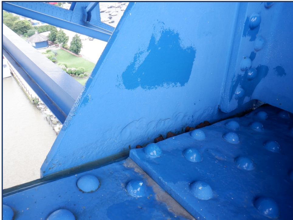
Photo 162-2 – Unit II, Span 8, North Truss, Painted over Section Loss on L23 Gusset Plate along Lower Chord
