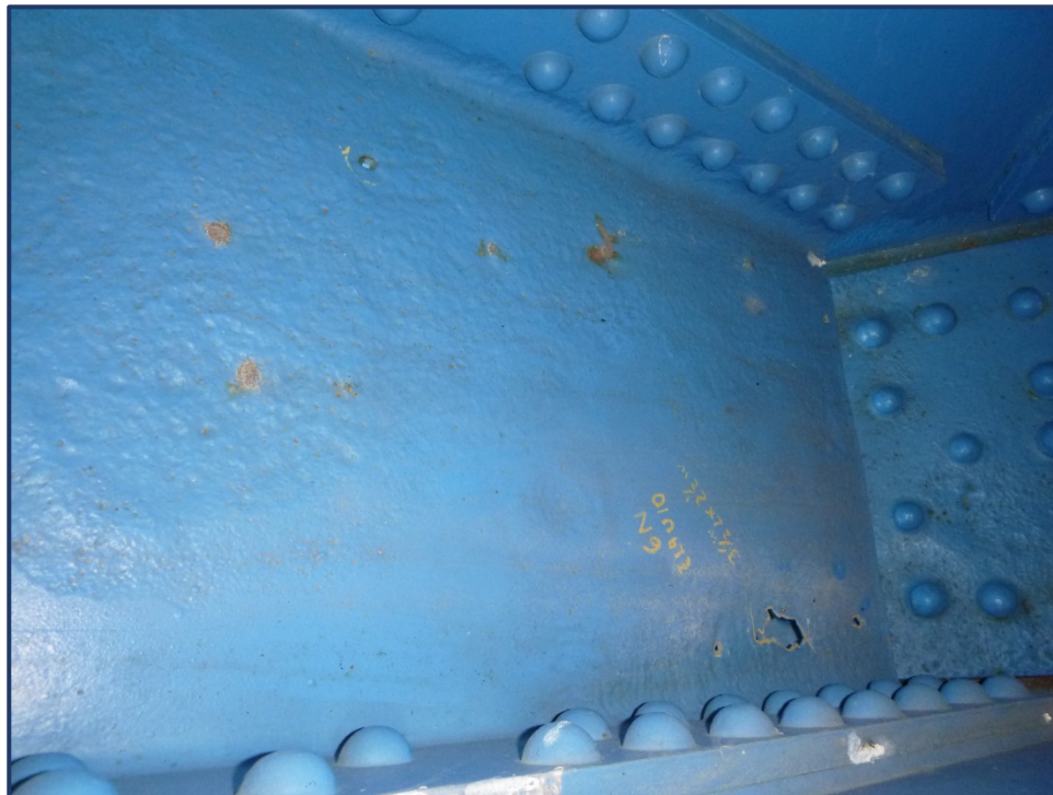
Photo 120-2 – Span 6, North Truss, Painted over Pitting and Corrosion Holes in Web of L9-U10 at L9
