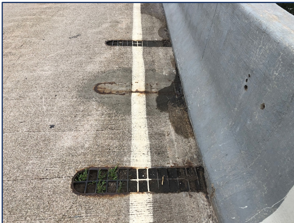
Photo 815-1 – Typical Clogged Scupper Inlets
