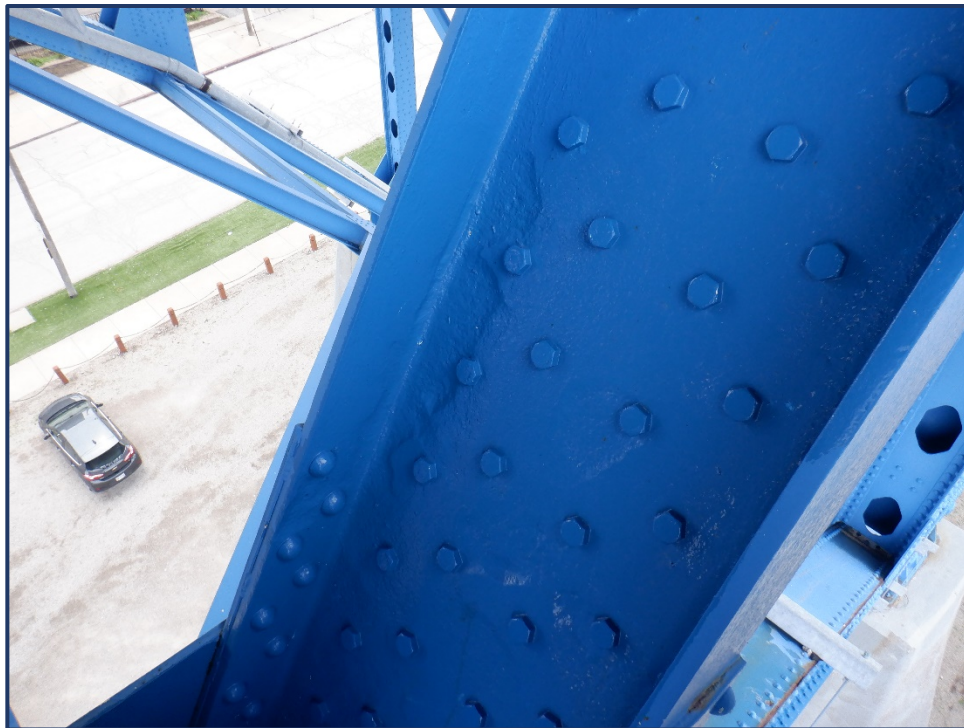
Photo 120-4 – Area of Painted over Section Loss on Diagonal with Retrofit Plate on Back Side
