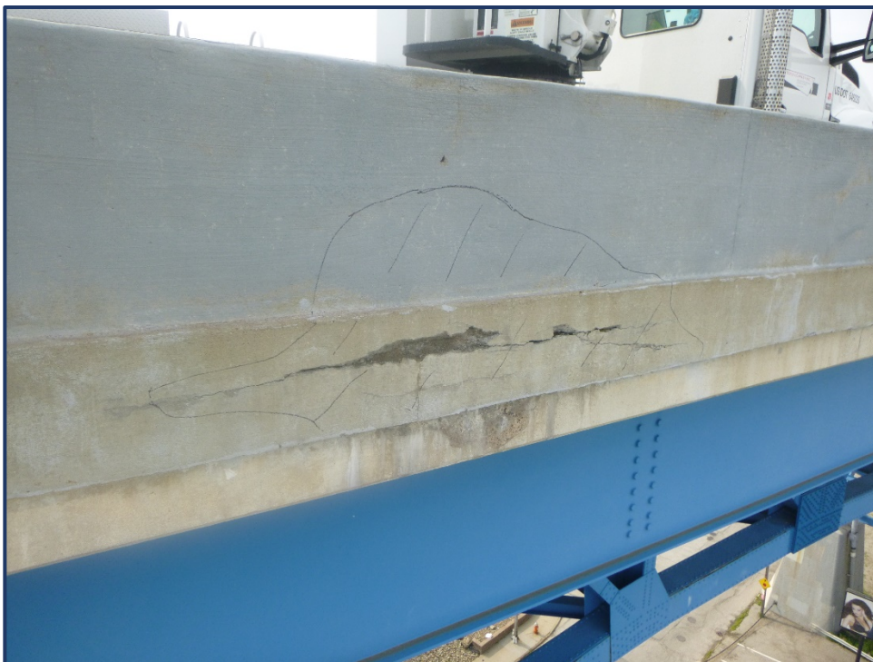
Photo 331-2 – Typical Area of Delamination & Spalling, Parapet Exterior Face
