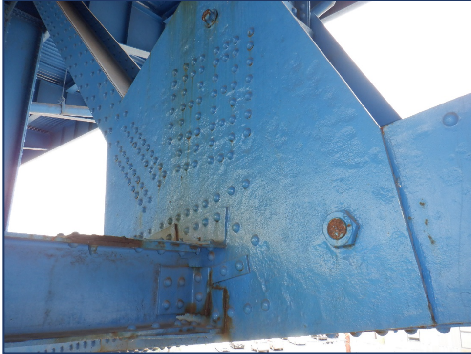
Photo 162-1 – Unit II, Span 1, South Truss, Painted Over Pitting on L7 Gusset Plate
