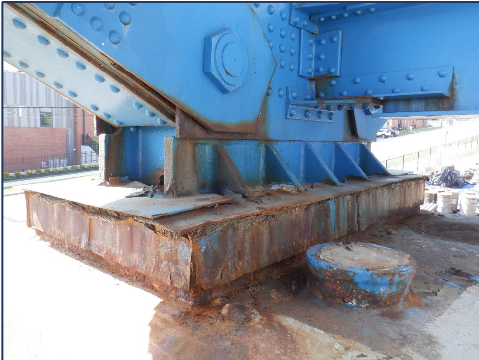
Photo 311-1 – Unit II, Pier 1, South Truss Bearing, Layered Corrosion
