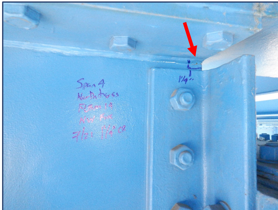
Photo 152-4 – Unit II, Span 4, FB 14 at North Truss, New Crack in Top Flange Cope
