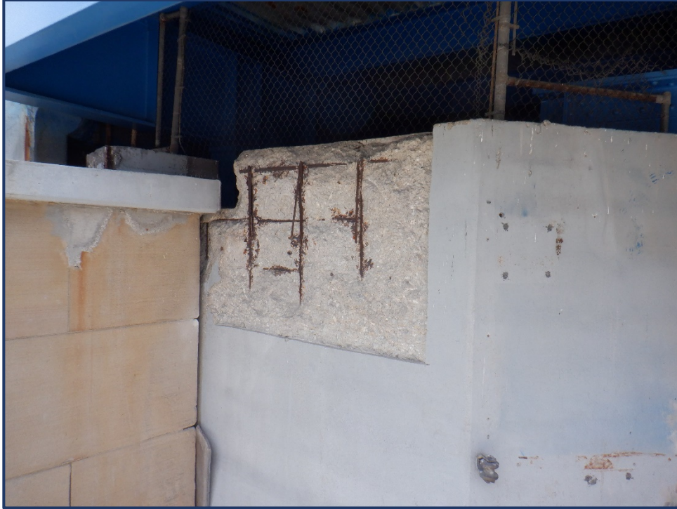
Photo MW-1 – Pier 37, Unit I, Section N, Spalling of Mask Wall at South Fascia
