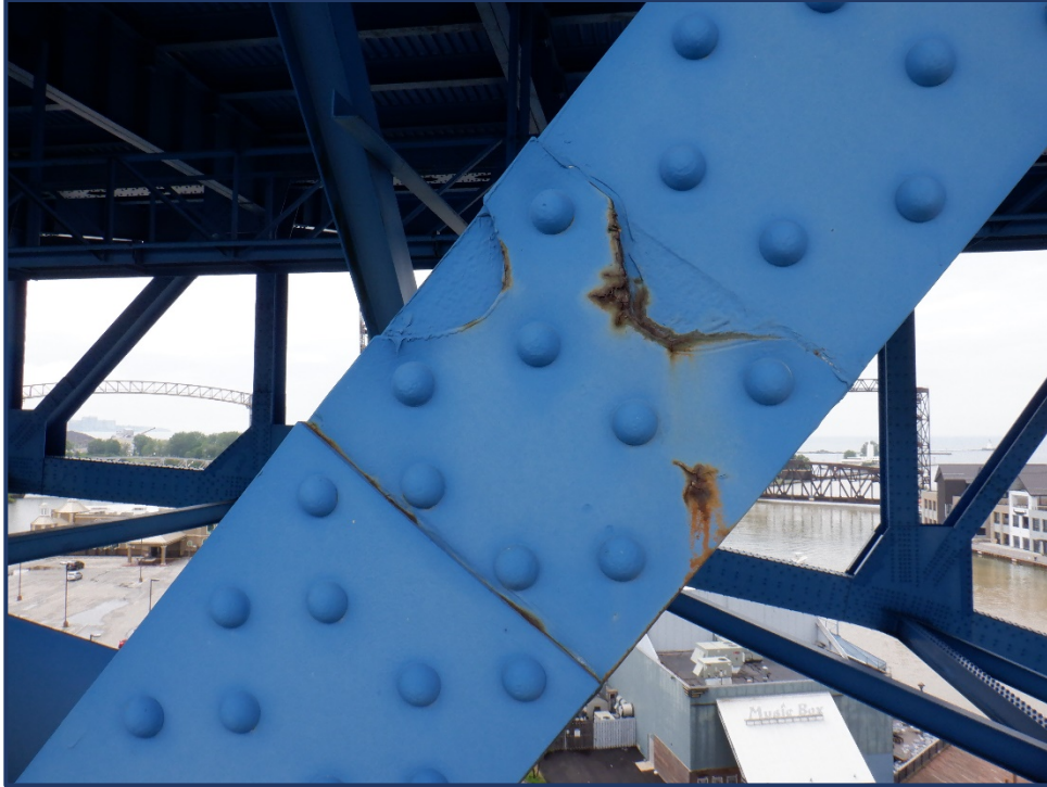
Photo 162-3 – Unit II, Span 8, South Truss, Corrosion Complete Section Loss In Fill Plate
