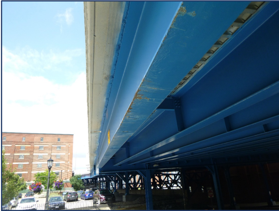
Photo 107-1 – Unit III, Bent 11-12, South Fascia Stringer, Vehicular Impact
