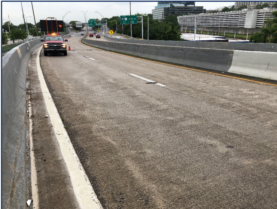
Photo AWS-1 – East Approach Pavement, Westbound Lanes, Areas of Asphalt Patching
