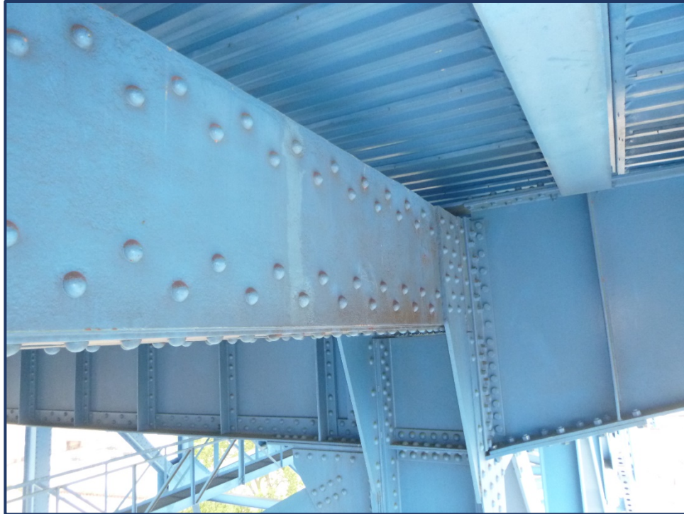
Photo 120-5 – Span 6, South Truss, U4-U5, Painted over Pitting and Web Plate Distortion
