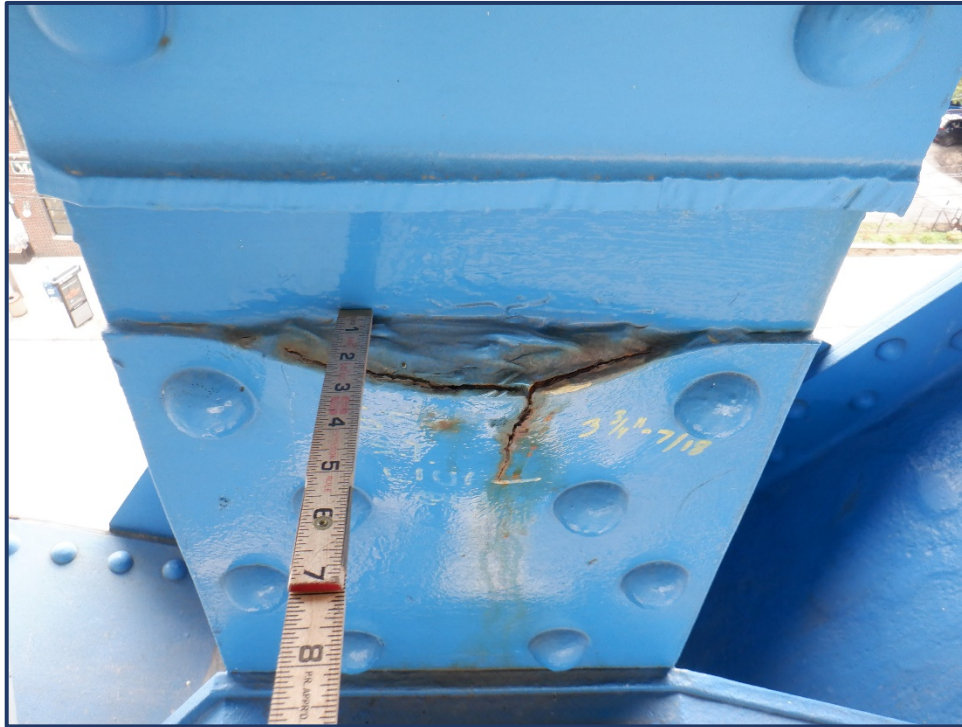
Photo 120-1 – Span 5, South Truss, Section Loss and Distortion due to Pack Rust at L1-U1 Fill Plate
