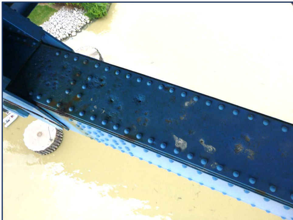
Photo 120-6 – Span 9, South Truss, L0-L1, Reactivating Section Loss
