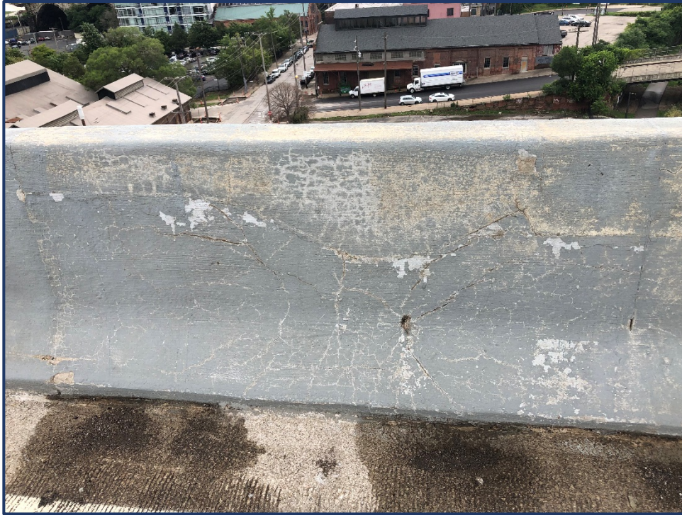
Photo 331-1 – Typical Area of Cracking, Parapet Interior Face
