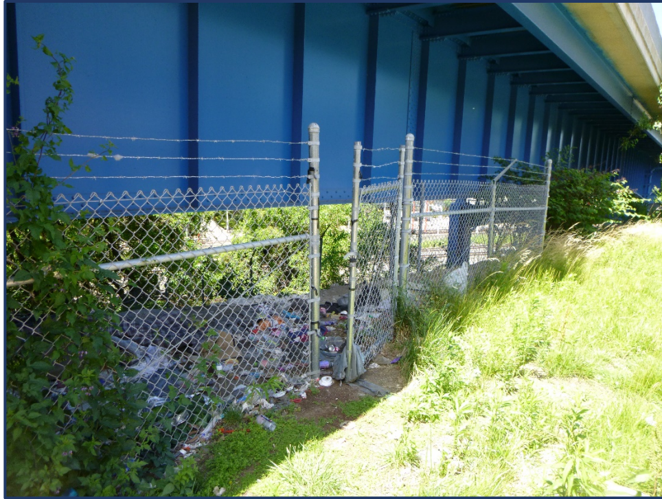
Photo APR-3 – Unit V, South Side of Pier 37, Open Vandal Fence Gate
