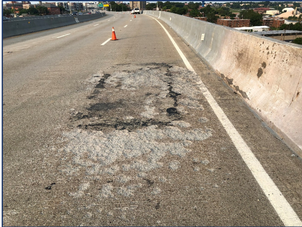
Photo 510-2 – Unit II, Span 6, Area of Shallow Spalling and Burn Marks in Westbound Lane 3
