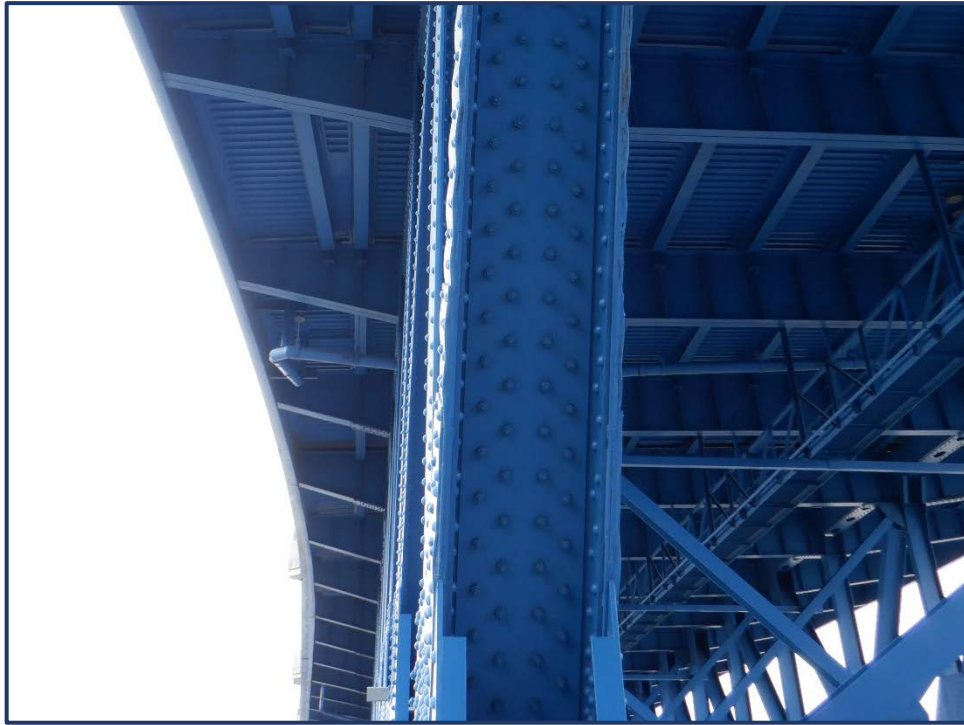
Photo 120-3 – Typical Distortion of Diagonal Flange Plates due to Sealed Pack Rust
