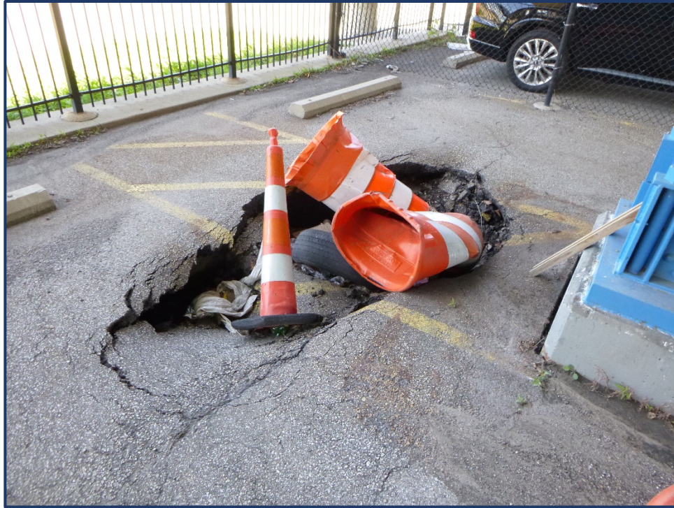
Photo APR-1 – Unit IV, Bent 30, Sinkhole in Parking Lot
