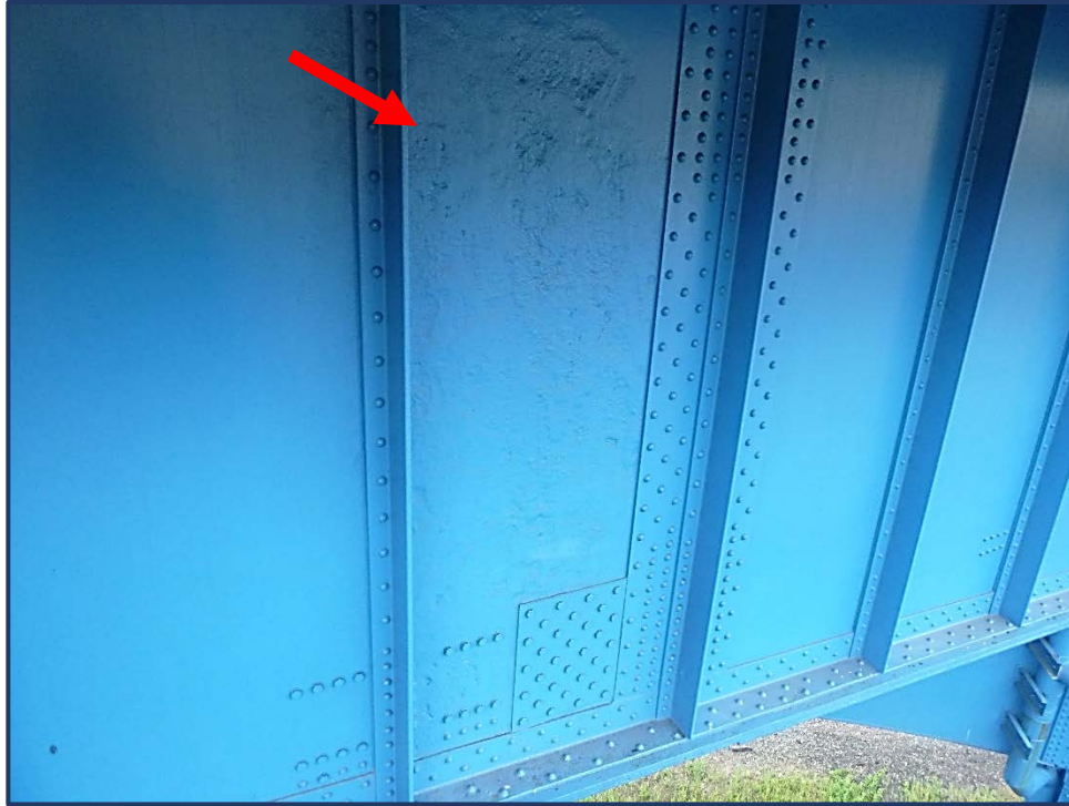
Photo 107-3 – Unit V, South Girder, ¼" Painted over Section Loss on Web
