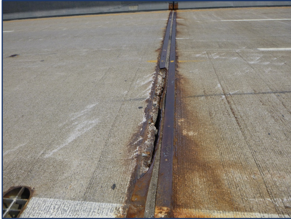
Photo 302-1 – Unit I, Joint X, 10-ft Section of Broken Retainer in Westbound Lane 3
