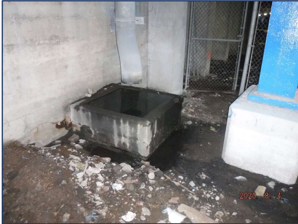
Photo 7 – Clogged catch basin at Joint R in Unit 1
