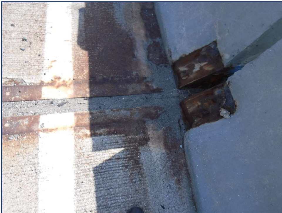
Photo 2 – Span J' Joint T Typical Rusting and Debris Impaction in Joints
