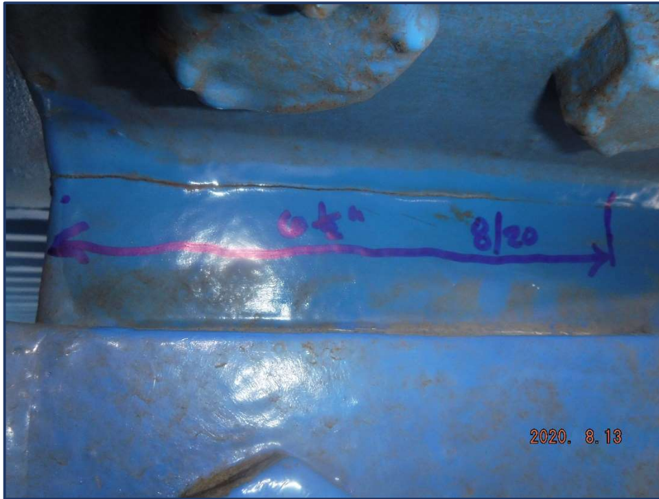
Photo 23 – 6½” long crack in east face top cope of Floorbeam 22 in Span 10
