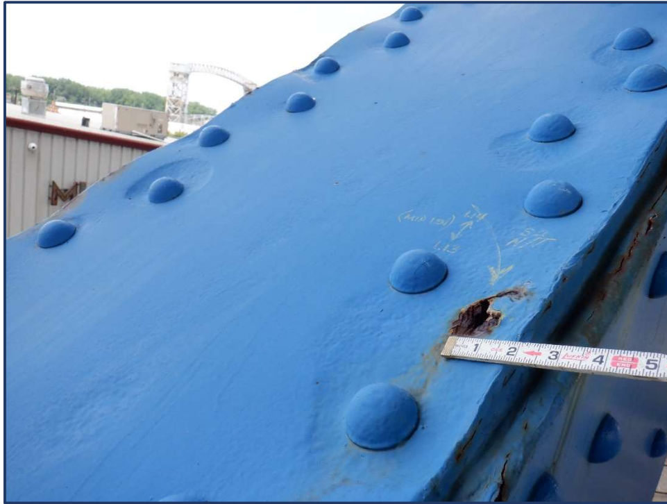
Photo 13 – 1" Diameter Corrosion Hole, L13L14, Span 2, North Truss
