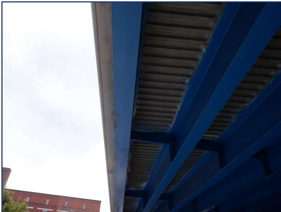
Photo 10 – South fascia beam over W. 9 th Street impact damage and impact scrapes on bottom flange
