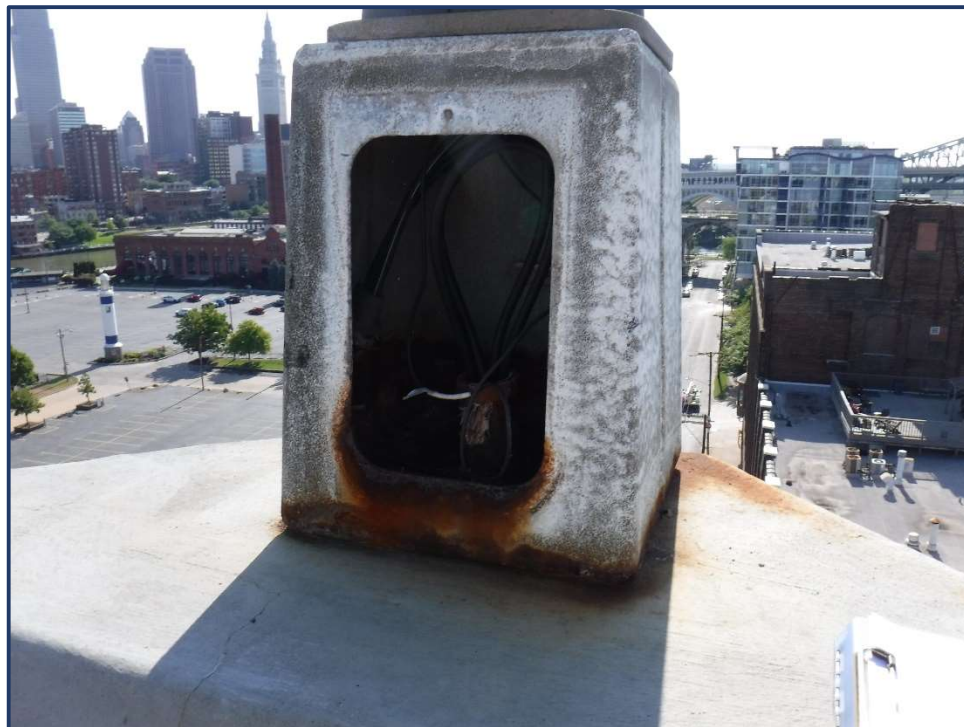
Photo 8 – Typical missing utility cover at light pole, Span 5 over Elm Street
