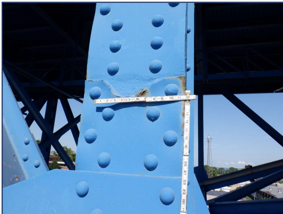
Photo 16 – 100% Section Loss in Fill Plate L15-U15, Span 2, South Truss
