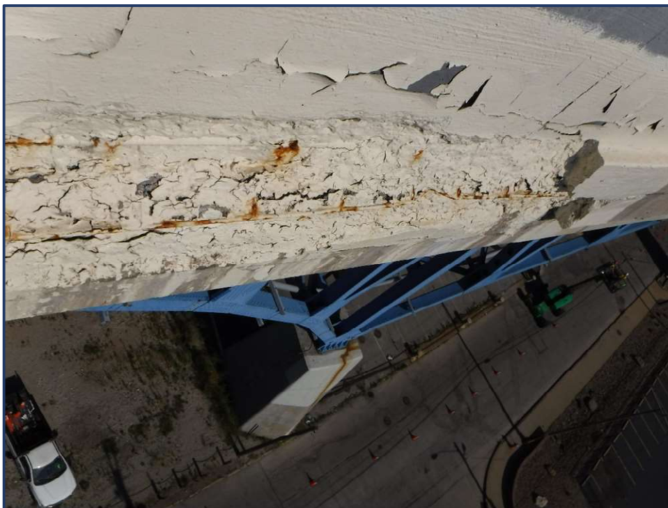
Photo 4 – Typical sealed spalls in exterior of parapet with corroded reinforcing South fascia west of Joint KC1 in Span 6 shown
