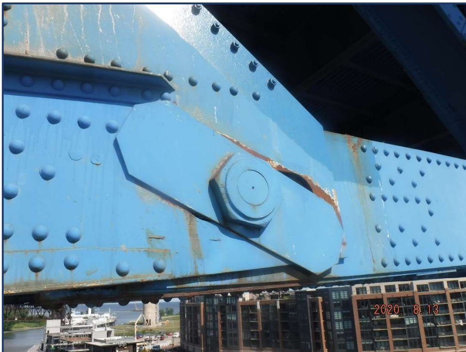
Photo 14 – Pin plate rotated, L0L1, Span 9, South Truss
