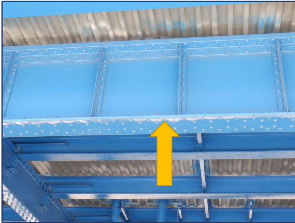
Photo 9 – 1" thick pack rust between bottom flange cover plate and flange. North girder over Lakeside Avenue shown
