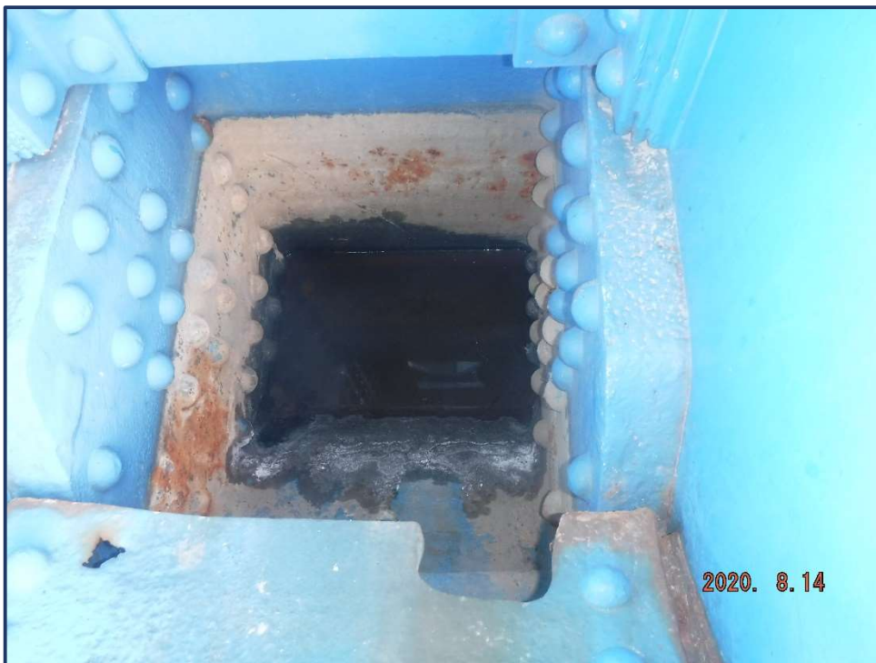
Photo 28 – Bearing assembly full of water, L1L2, Span 4, South Truss
