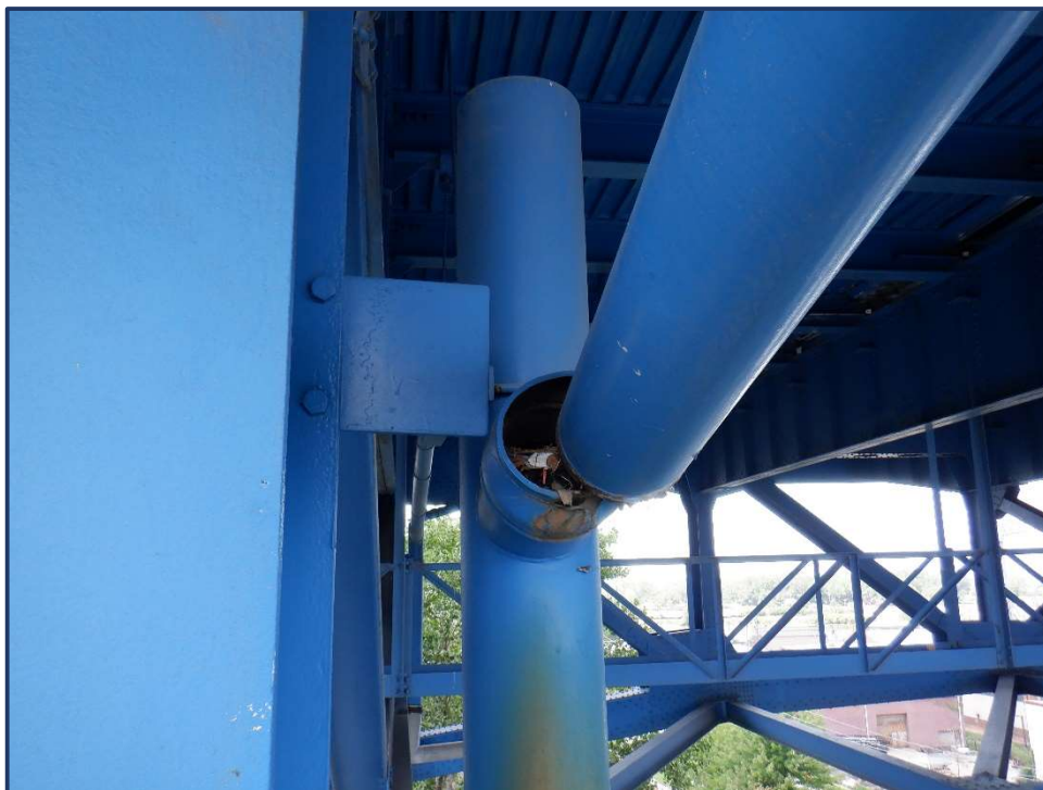
Photo 6 – Broken Downspout at South Truss L6U6 in Span 2
