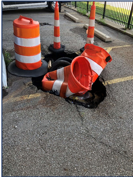
Photo 31 – 6' diameter x 4' deep sink hole in parking lot at Bent 30
