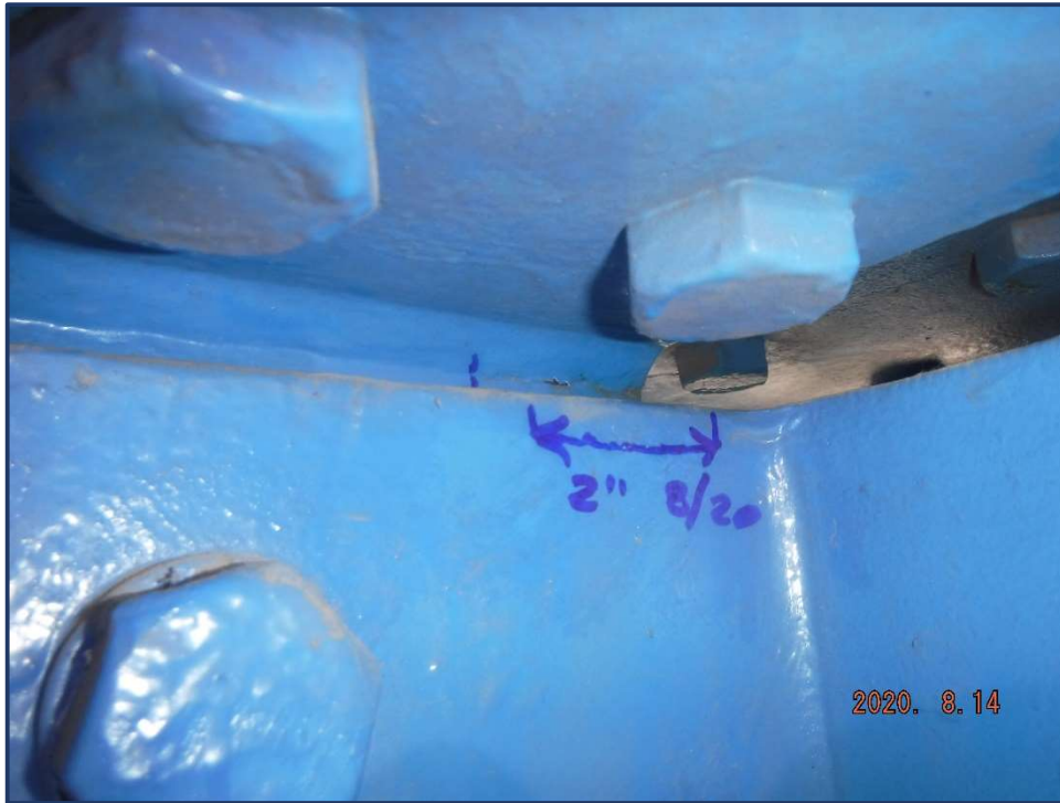
Photo 21 – 2" long crack in east face of top cope of Floorbeam 0 in Span 6
