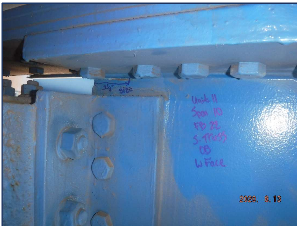
Photo 26 – 3/4" long crack west face outboard top cope of FLBM 22 Span 10
