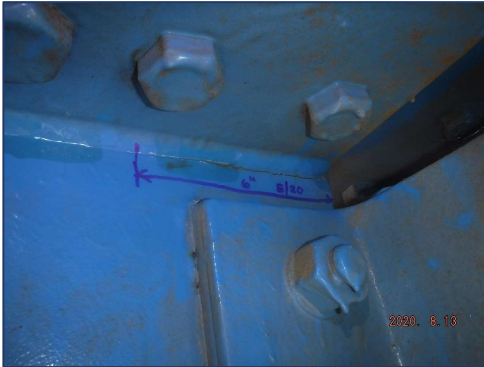
Photo 25 – 6" long crack east face outboard top cope of FLBM 22 in Span 10
