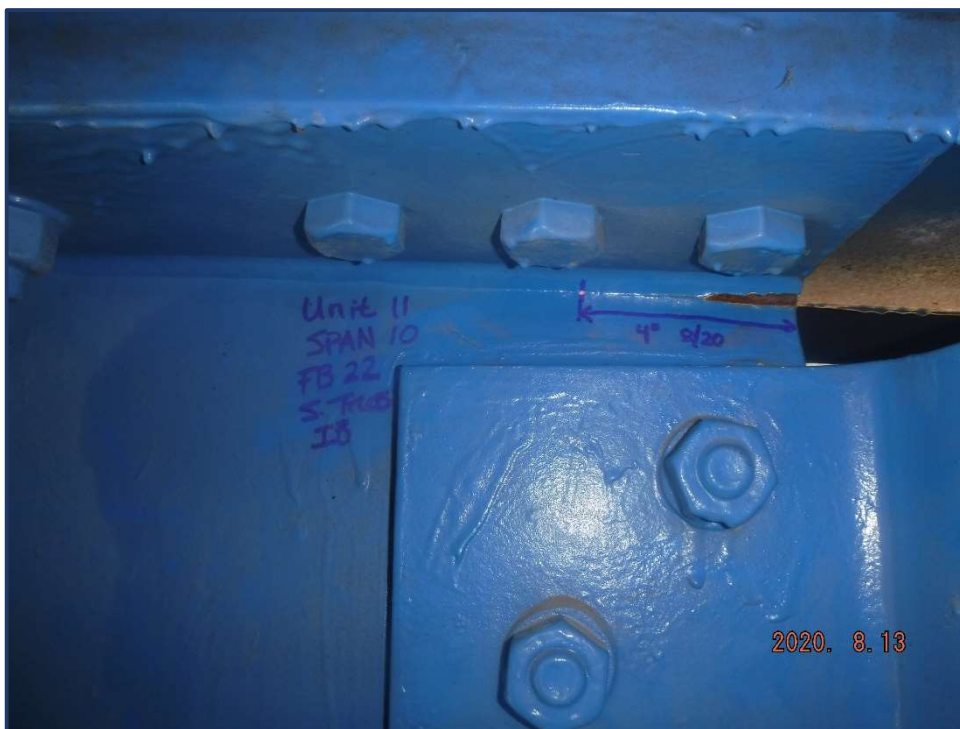
Photo 24 – 4” long crack in east face top cope of Floorbeam 22 in Span 10
