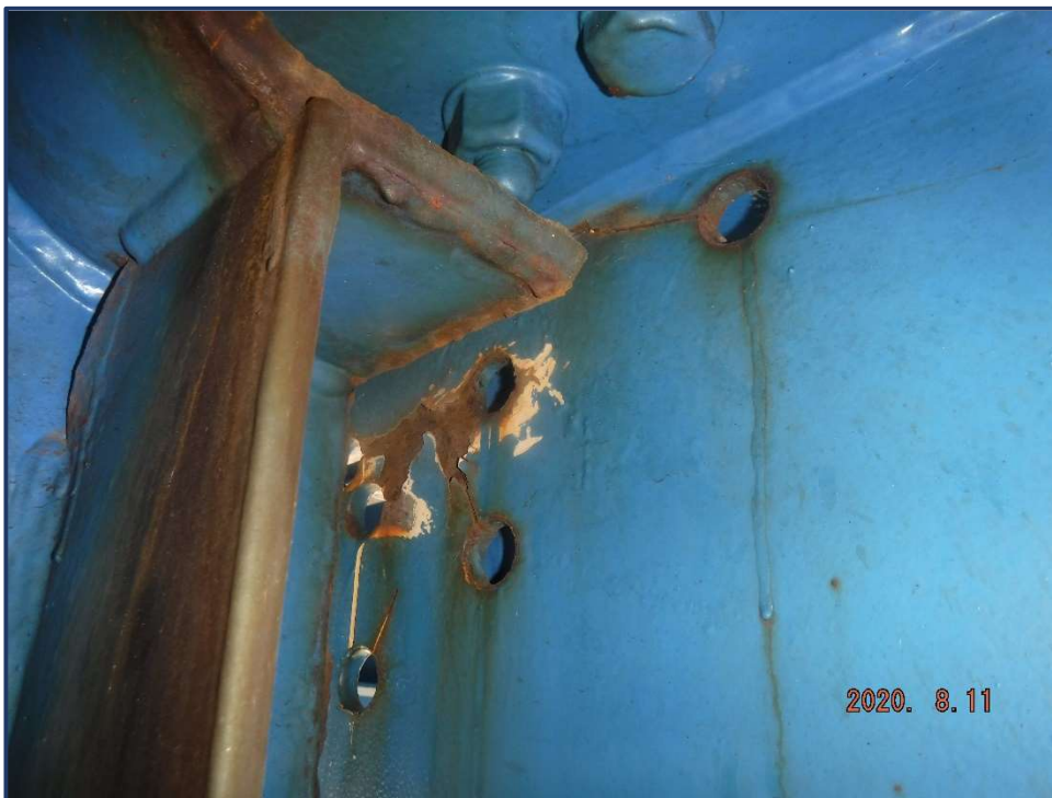
Photo 18 – Span 8, Floorbeam 25 Fatigue Cracks with Arrest Holes
