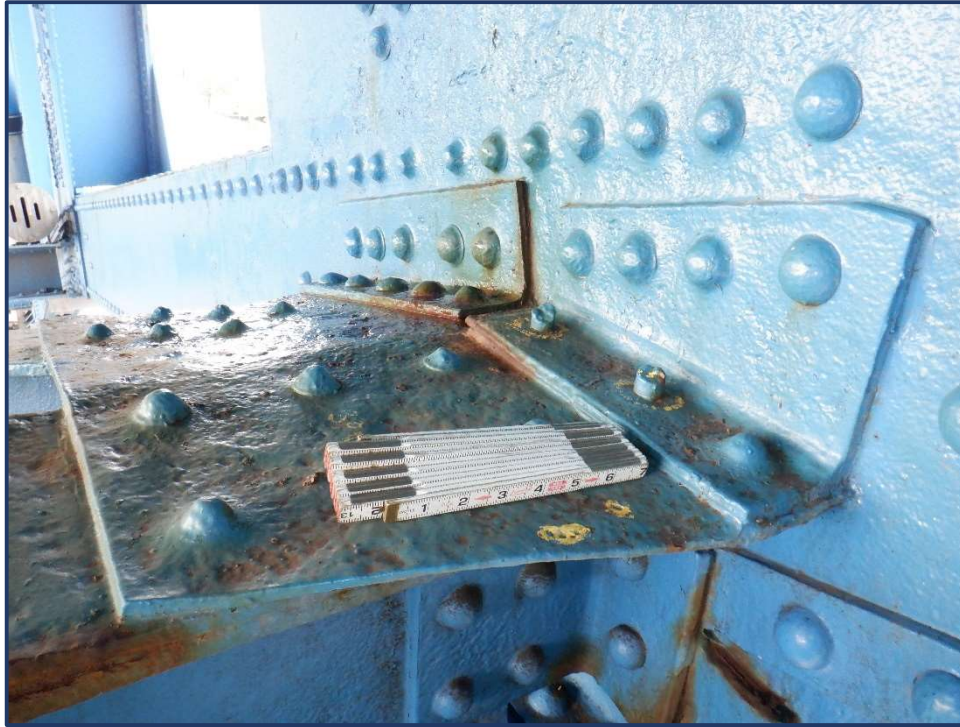
Photo 17 – Lower Lateral Bracing Gusset Defects, L7, Span 1, South Truss
