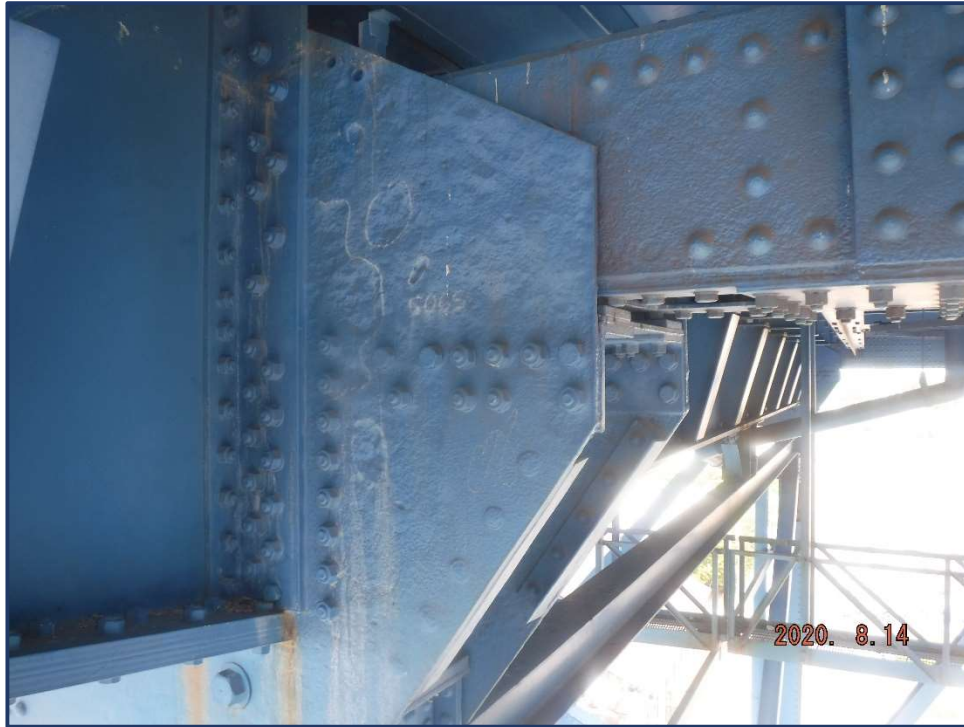
Photo 15 – Up to ¼” deep pitting in pin plate, U0, Span 6, South Truss
