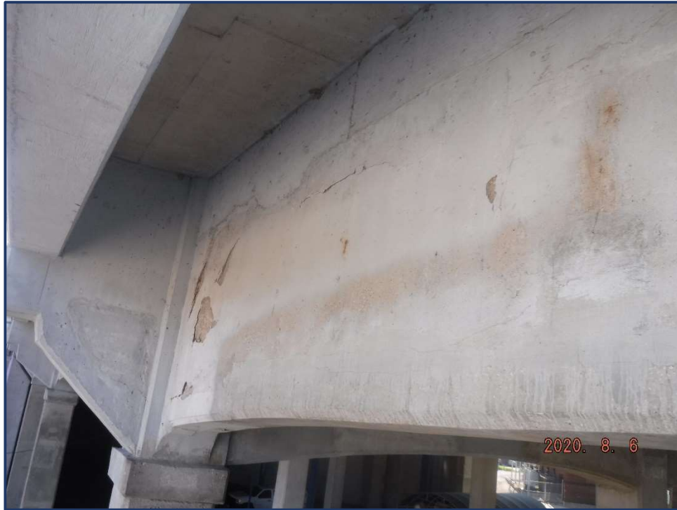
Photo 11 – 12' long x 4' high delaminated area in Girder 15 in Section P
