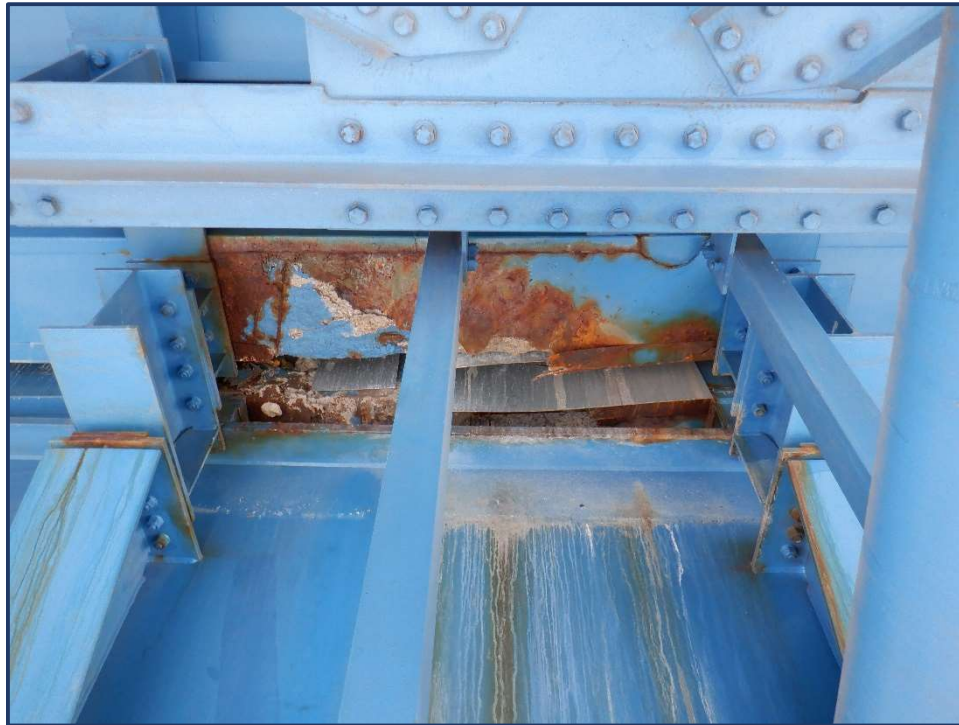
Photo 3 – Joint L Header Spalled and Delaminated Concrete
