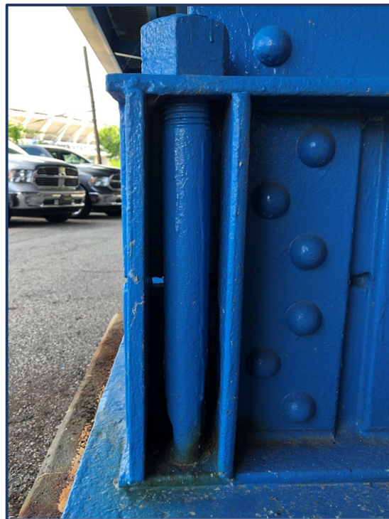
Photo 30 – Typical painted over section loss in anchor bolts, Bent 34, Unit IV
