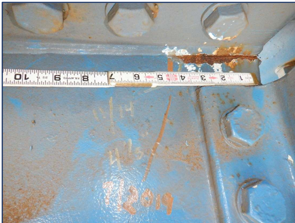
Photo 20 – Span 1, FLBM 7 South Cantilever 5½” Long Crack at Top Flange
