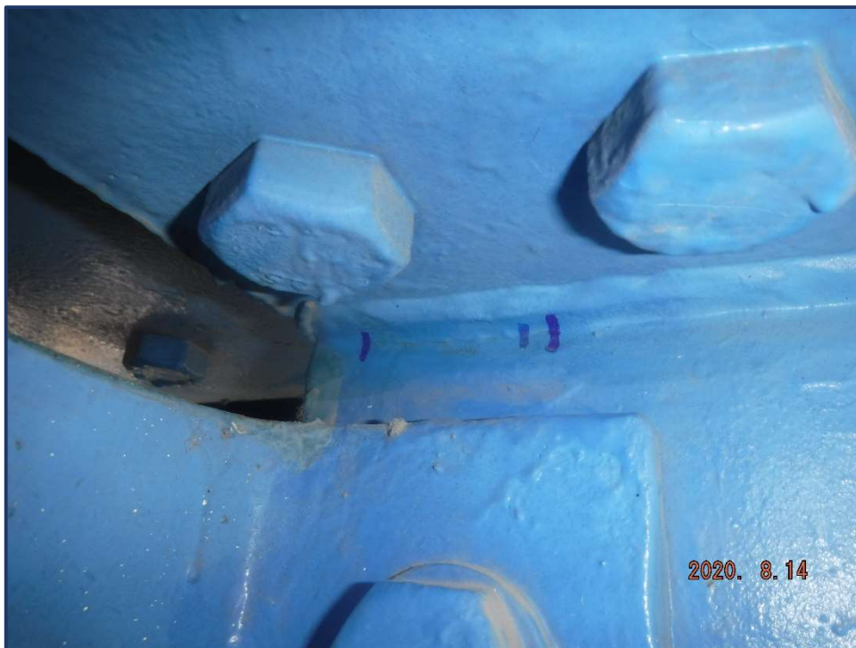
Photo 22 – 2 1/8" long crack in west face of top cope of Floorbeam 0 in Span 6
