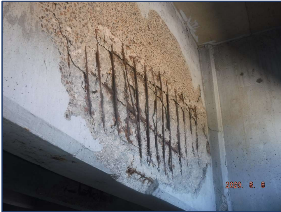
Photo 27 – 7' long x 4' high x 3" deep spall with exposed rebar with 100% section log, Floorbeam 0 west cantilever, south face, Section P,
