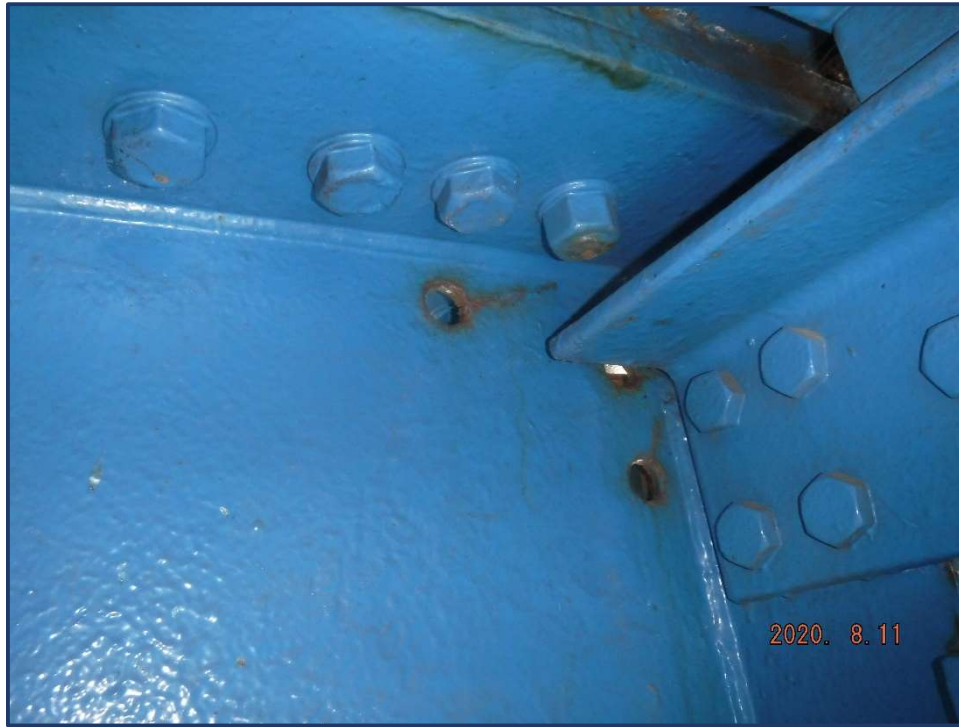
Photo 19 – Span 8, Floorbeam 25 North Cantilever Arrested Fatigue Cracks
