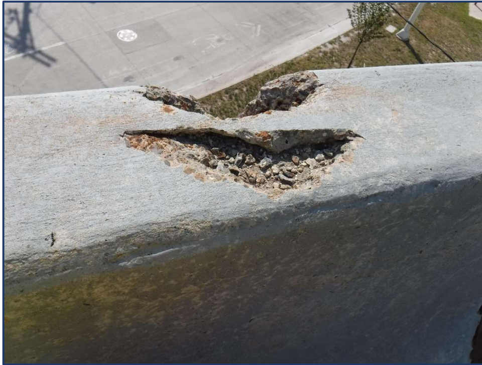
Photo 5 – Spalled parapet in Section N near Joint Q
