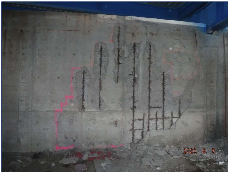
Photo 32 – Spall with exposed rebar in north wall of south vault at W. 9 th Street
