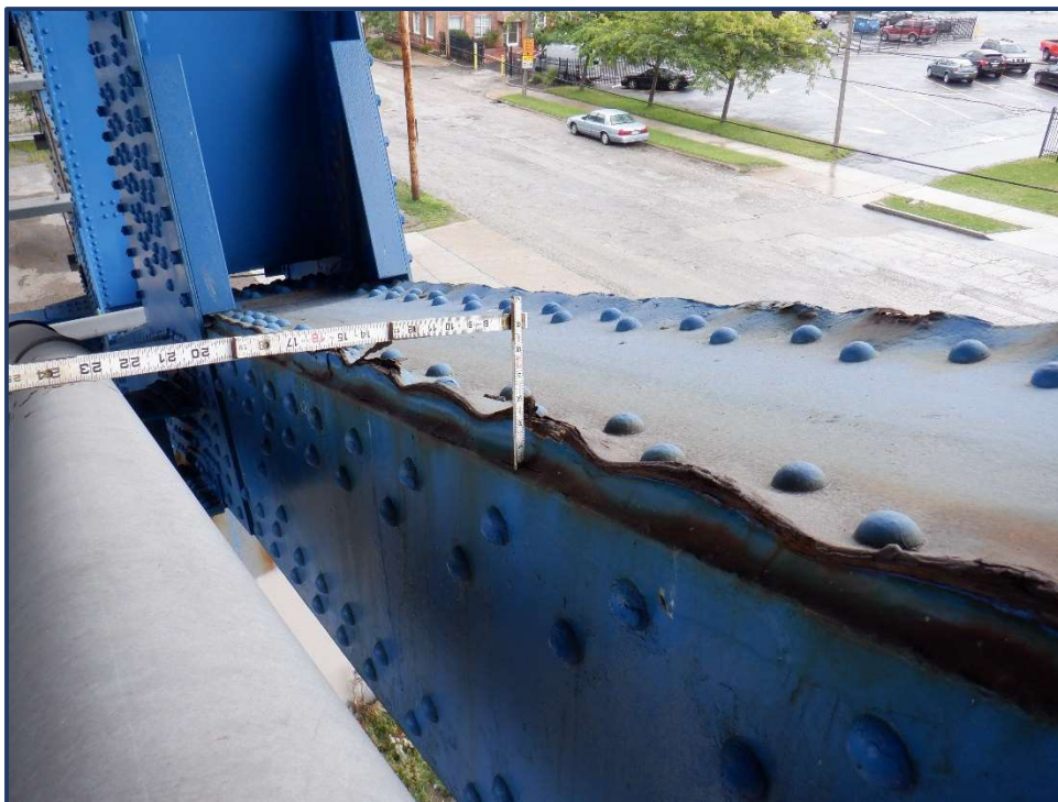
Photo 12 – Pack Rust Induced Distortion in Lower Chord L1L2, Span 2, South Truss
