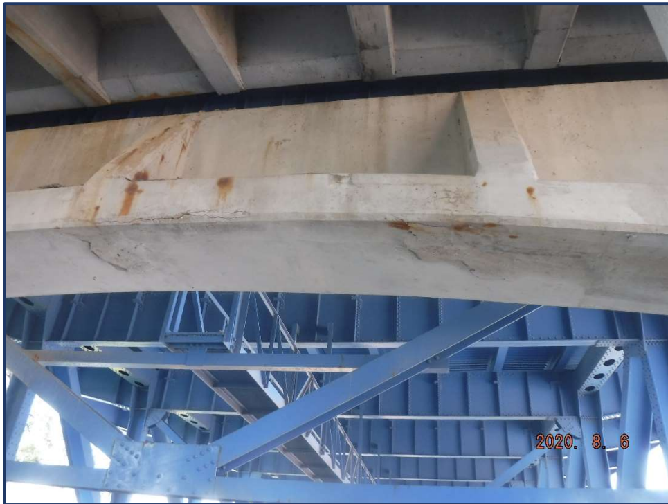
Photo 29 – Delaminated Areas in Pier O Cap
