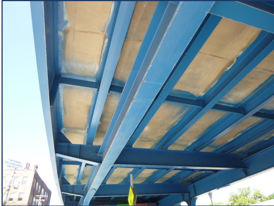
Photo 107-1 – Unit II, over W 28 th Street, South Fascia Girder, Vehicular Impact
