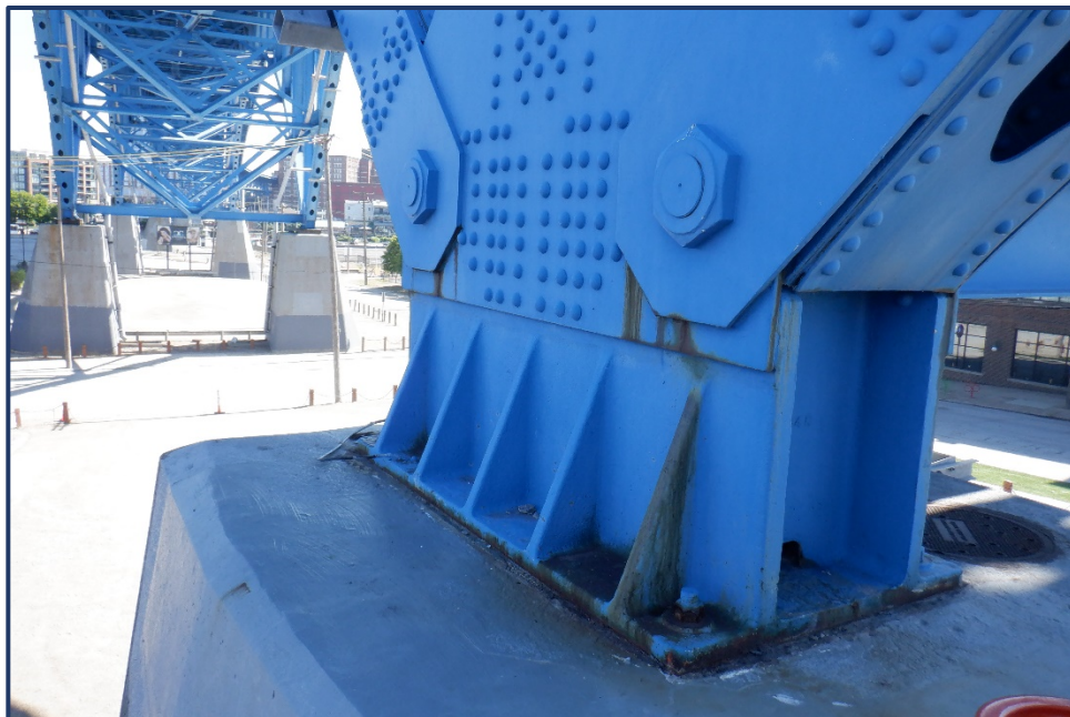
Photo 313-1 – Unit II, Pier 4, North Truss Bearing, Section Loss of Bearing and Anchor Bolt Nuts
