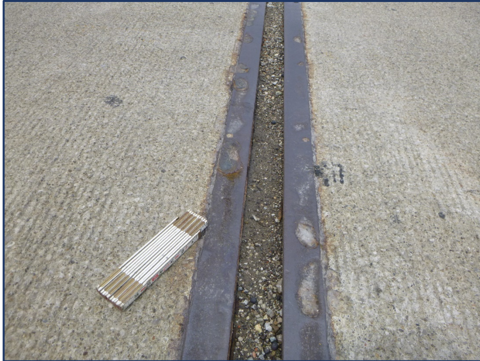
Photo 302-1 – Typical Debris Impaction and Section Loss in Compression Seal Joints
