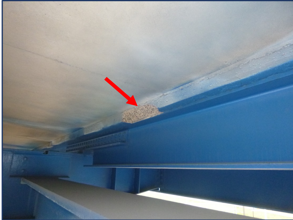
Photo 12-1 – Scattered Haunch Spalling in Unit I
