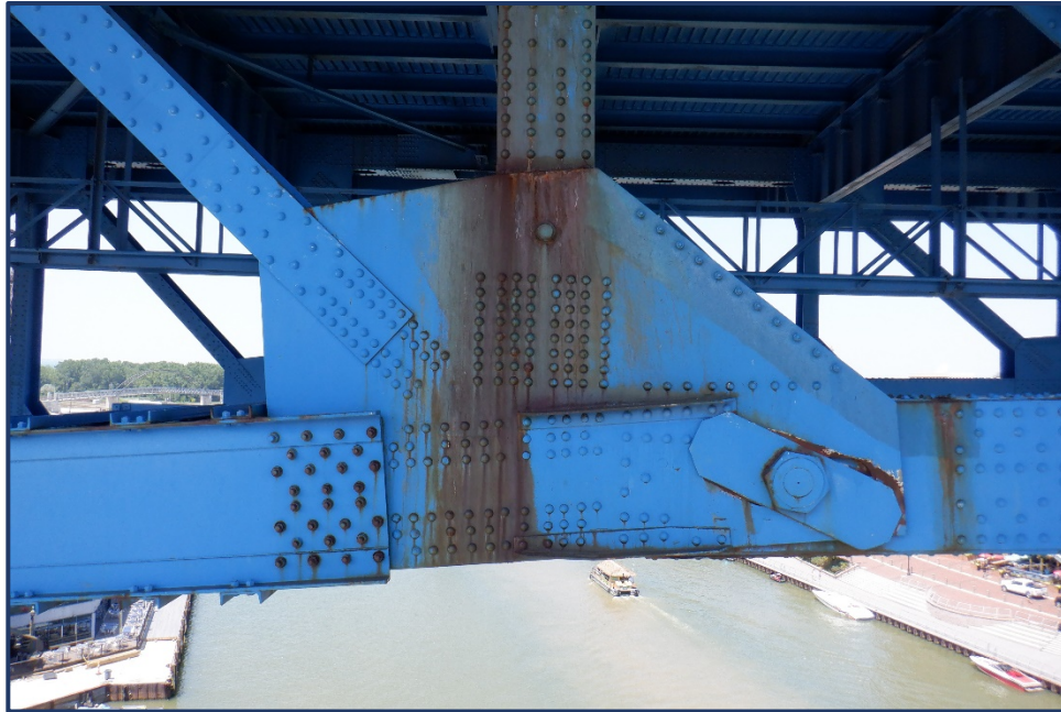
Photo 161-2 – Unit II, Span 9, South Truss, Rotated Pin Plate at L0
