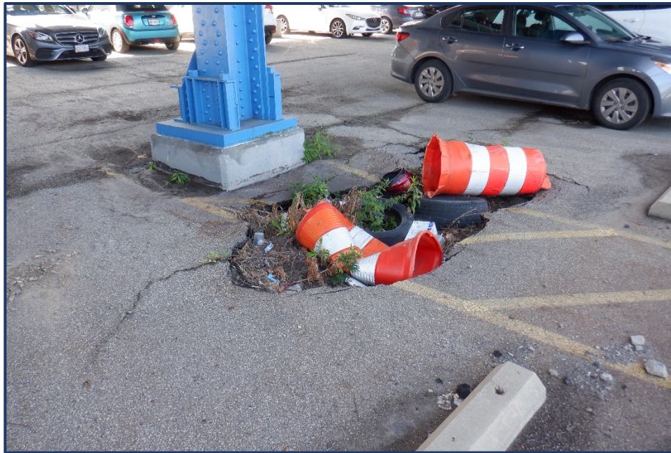
Photo APR-1 – Unit IV, Bent 30, Sinkhole in Parking Lot
