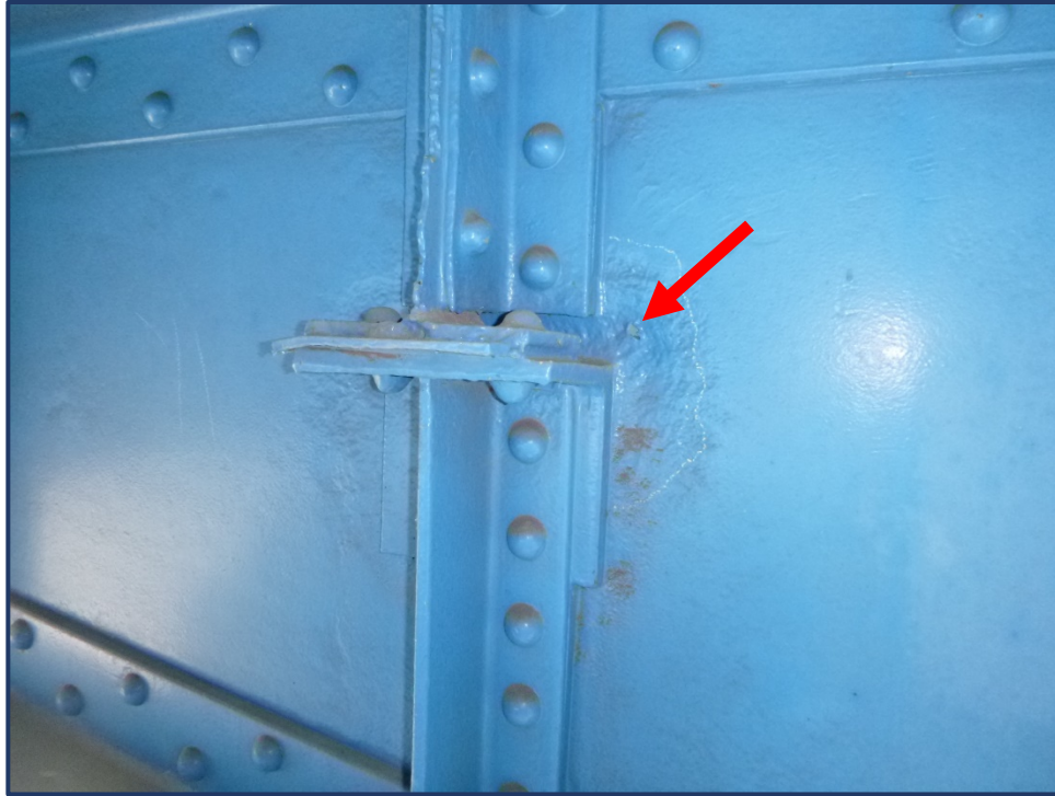
Photo 152-3 – Unit II, Span 10, FB 16, Areas of Painted over Section Loss with Corrosion Holes at Abandoned Stringer Connection
