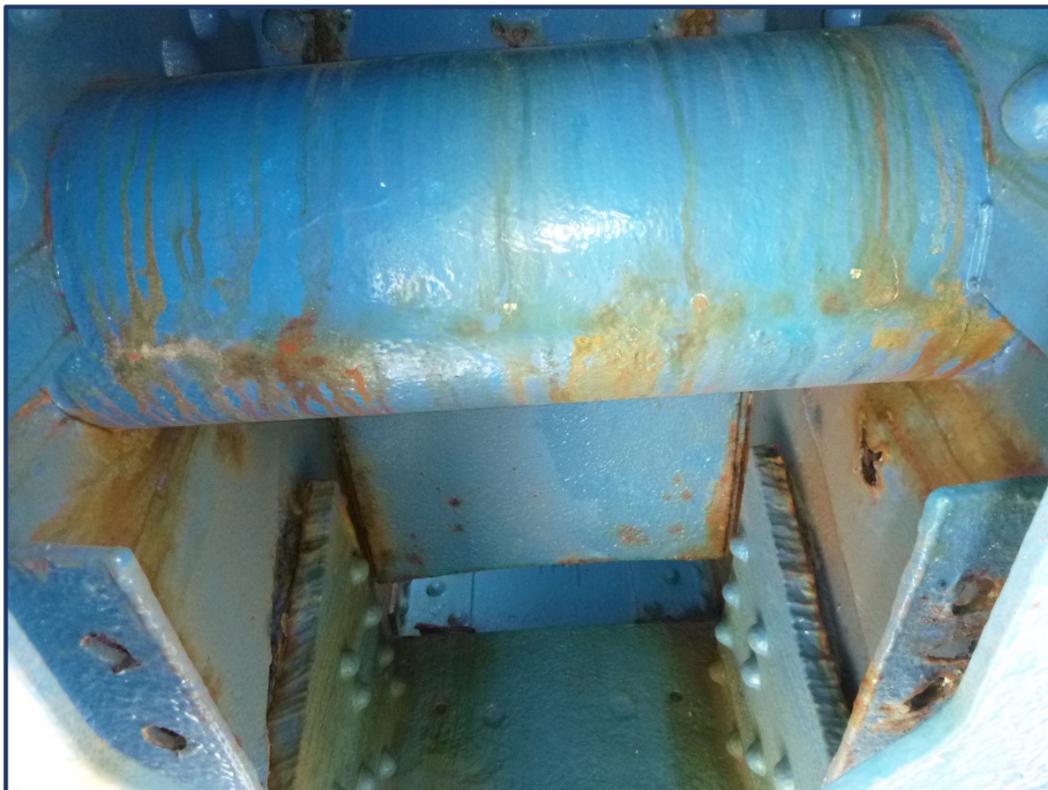
Photo 161-1 – Unit II, Span 8, North Truss at U25, Painted over Pitting on Pin with Rust Staining
