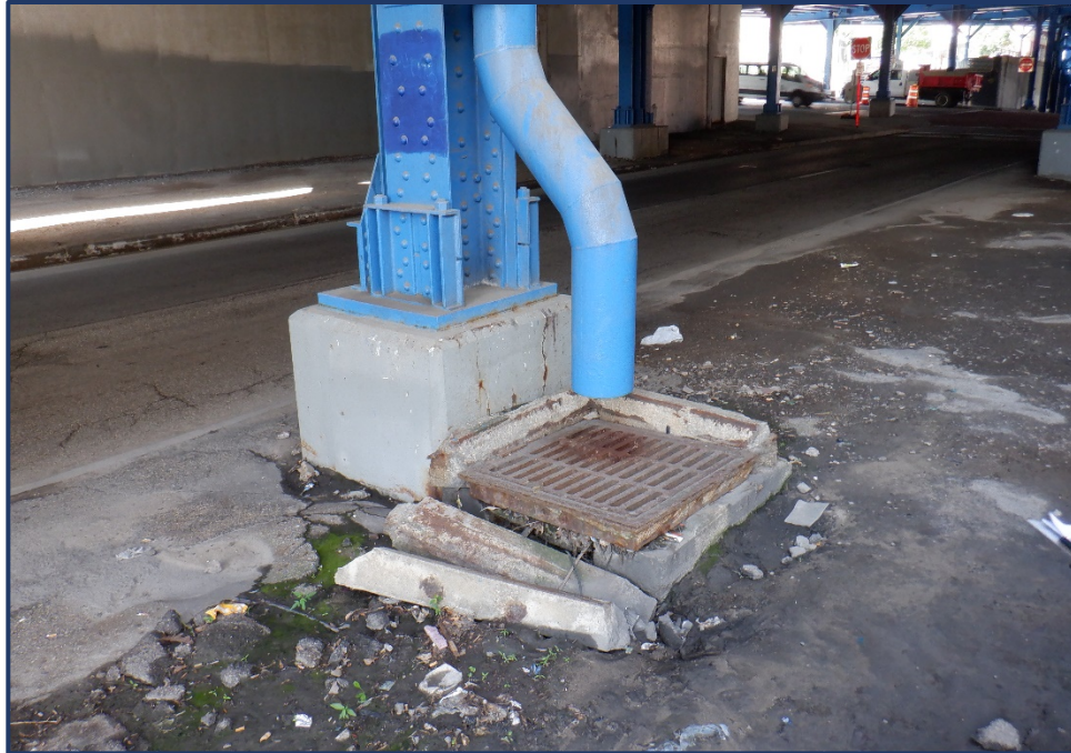
Photo 815-2 – Unit IV, Bent 15 Catch Basin, Heavy Spalling of Frame and Shifting Grate
