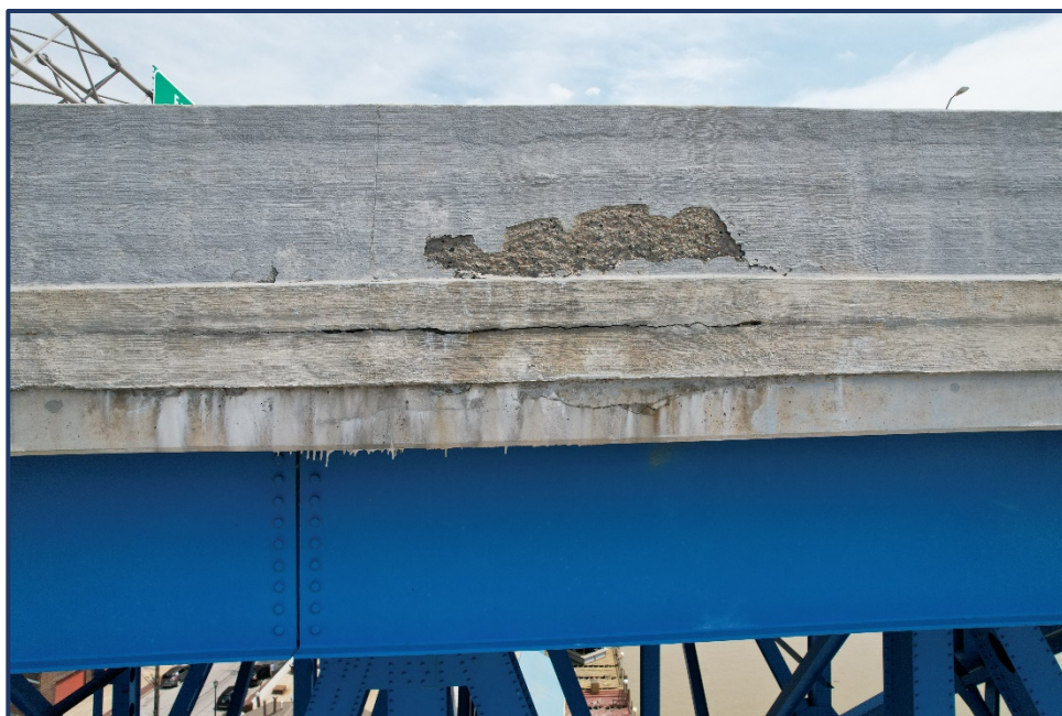
Photo 331-2 – Typical Area of Delamination & Spalling, Parapet Exterior Face
