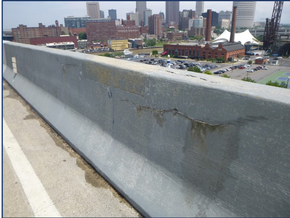
Photo 331-1 – Typical Area of Cracking, Parapet Interior Face
