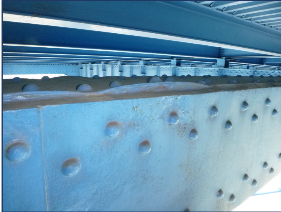
Photo 120-5 – Span 6, South Truss, U14-U15, Painted over Pack Rust
