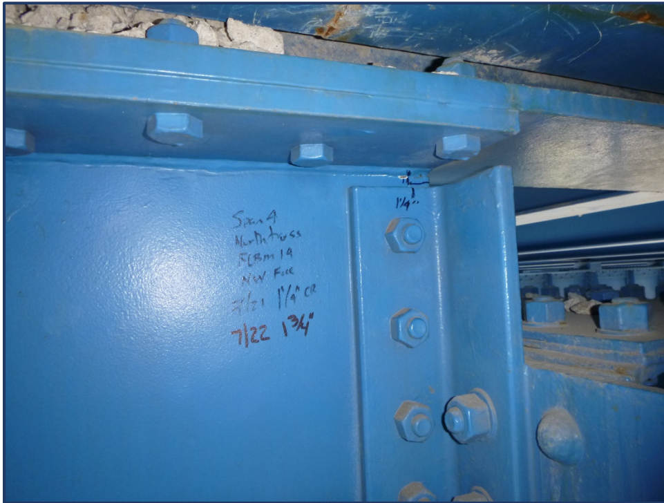
Photo 152-5 – Unit II, Span 4, FB 14 at North Truss, Crack in OB Top Flange Cope Exhibiting Slow Growth
