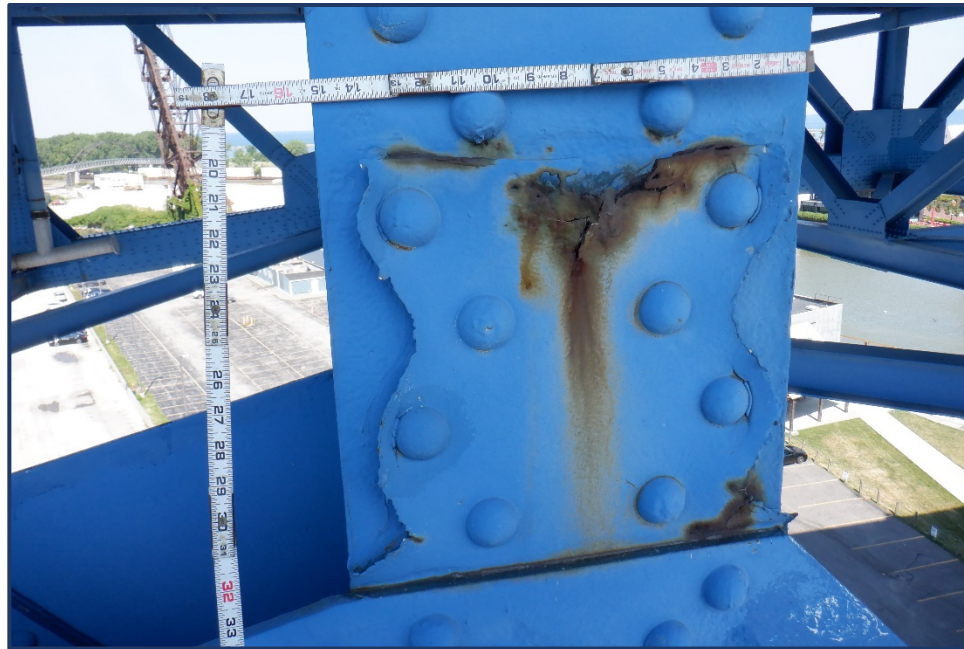
Photo 162-3 – Unit II, Span 8, North Truss, Corrosion Complete Section Loss In Fill Plate at L9
