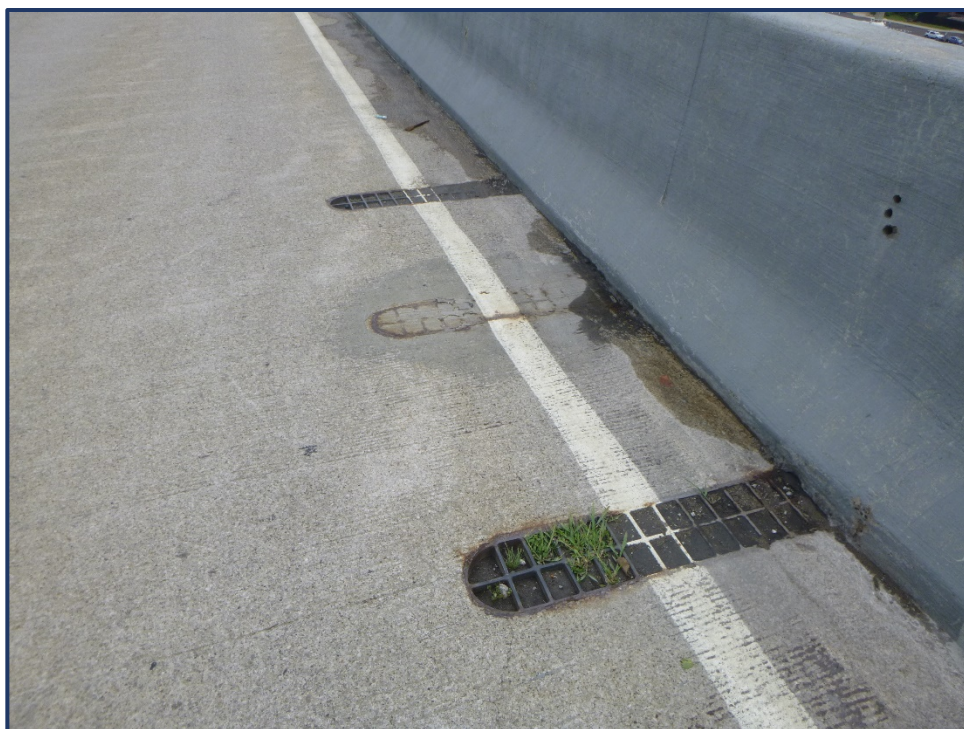
Photo 815-1 – Typical Clogged Scupper Inlets
