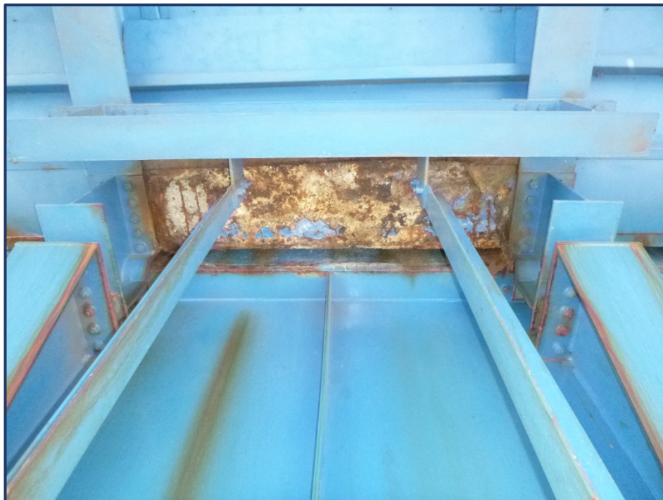
Photo 303-2 – Unit II, Joint J Header Spalled and Delaminated Concrete
