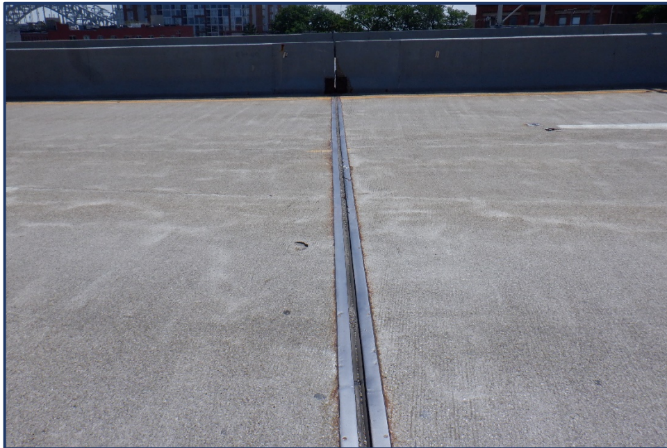
Photo 300-1 – Typical Debris Impaction and Impact Damage in Strip Seal Joints
