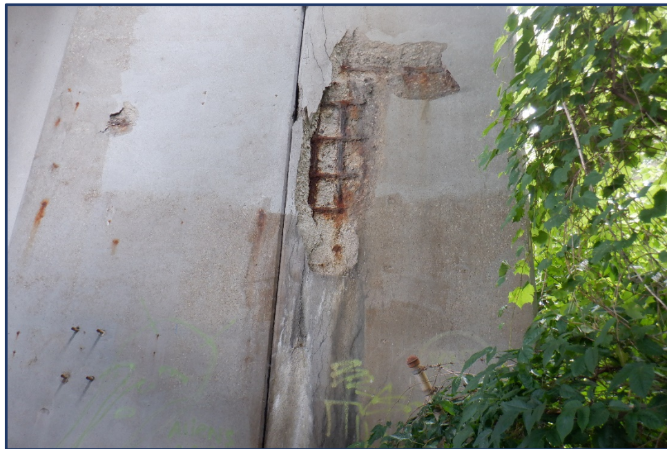
Photo 205-1 – Unit I, Section P, East Pier, Spalling of North Column
