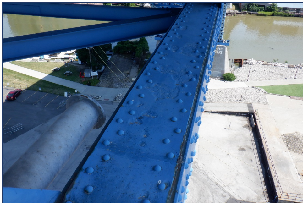
Photo 120-6 – Span 8, South Truss, L8-L9, Painted over Section Loss
