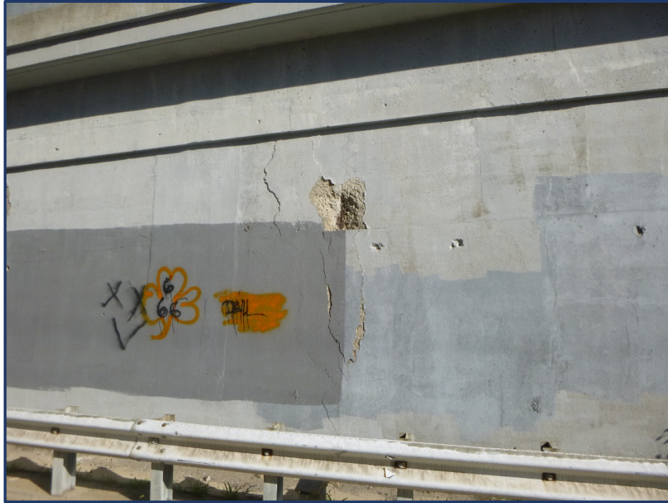
Photo MW-1 – Unit I, Section J', Spalling and Delamination in South Mask Wall
