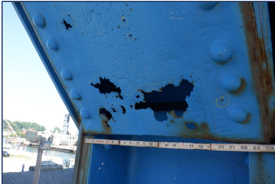
Photo 120-8 – Span 4, South Truss, L1-L2, Painted over Corrosion Holes in Bottom Flange
