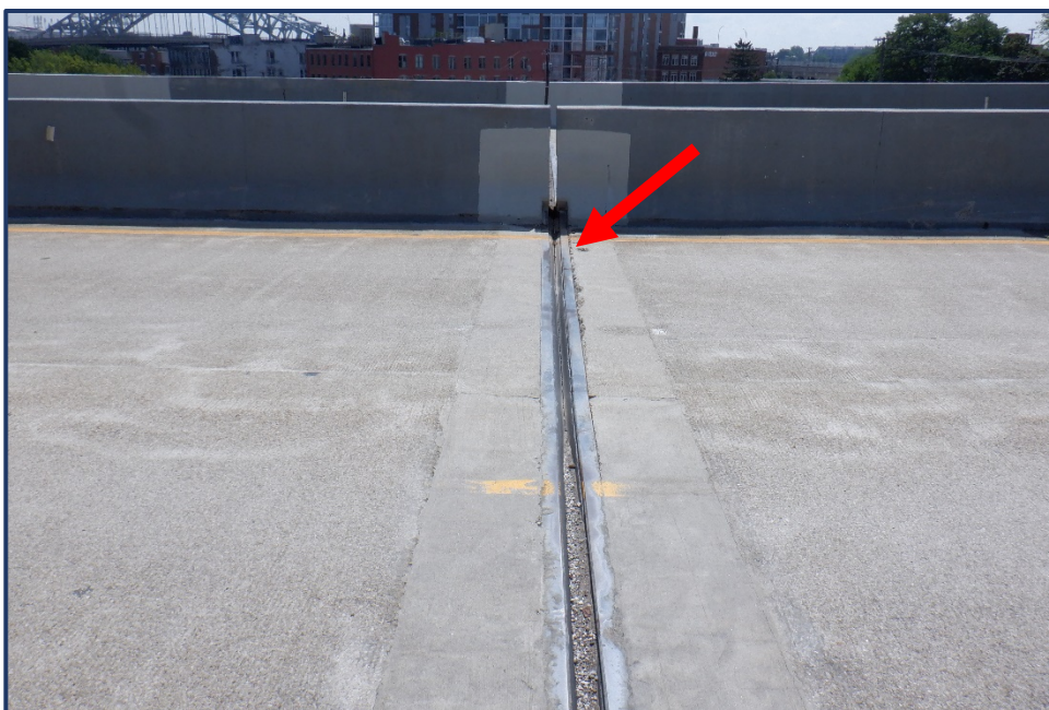
Photo 300-2 – Joint O Loose Joint Armor and Spalled
