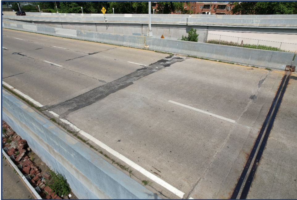
Photo 321-1 – West Approach Slab, Eastbound, Areas of Asphalt Patching in Approach Slab and Joint.
