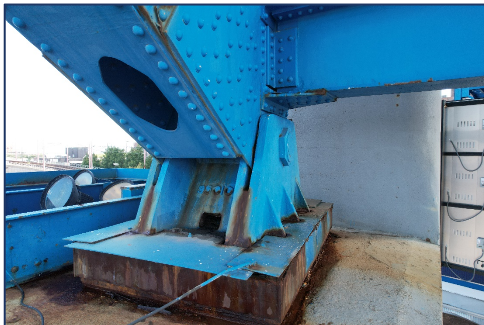
Photo 311-1 – Unit II, Pier 10, North Truss Bearing, Layered Corrosion
