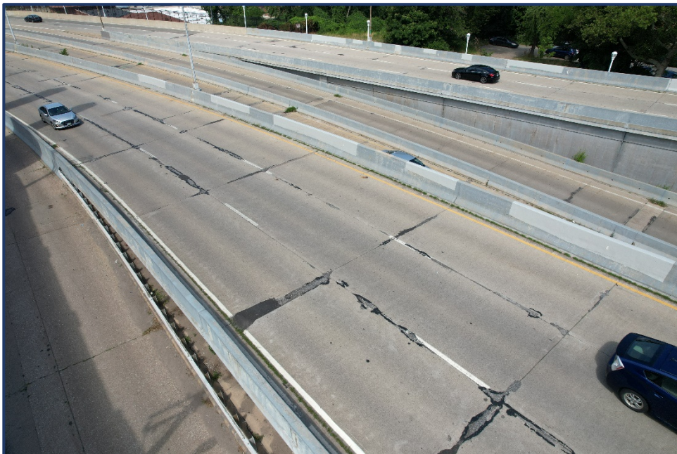
Photo AWS-1 – West Approach Pavement, Westbound, Areas of Potholes and Asphalt Patching
