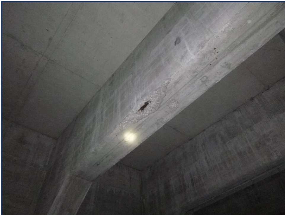
Photo 234-1 – Unit I, Pier 12 Cap, Spall with Exposed Reinforcing
