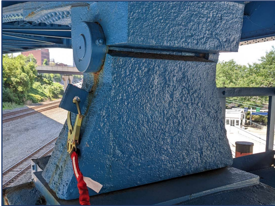
Photo 311-2 – Unit V, Pier 39, Center Bearing, Painted Over Pitting
