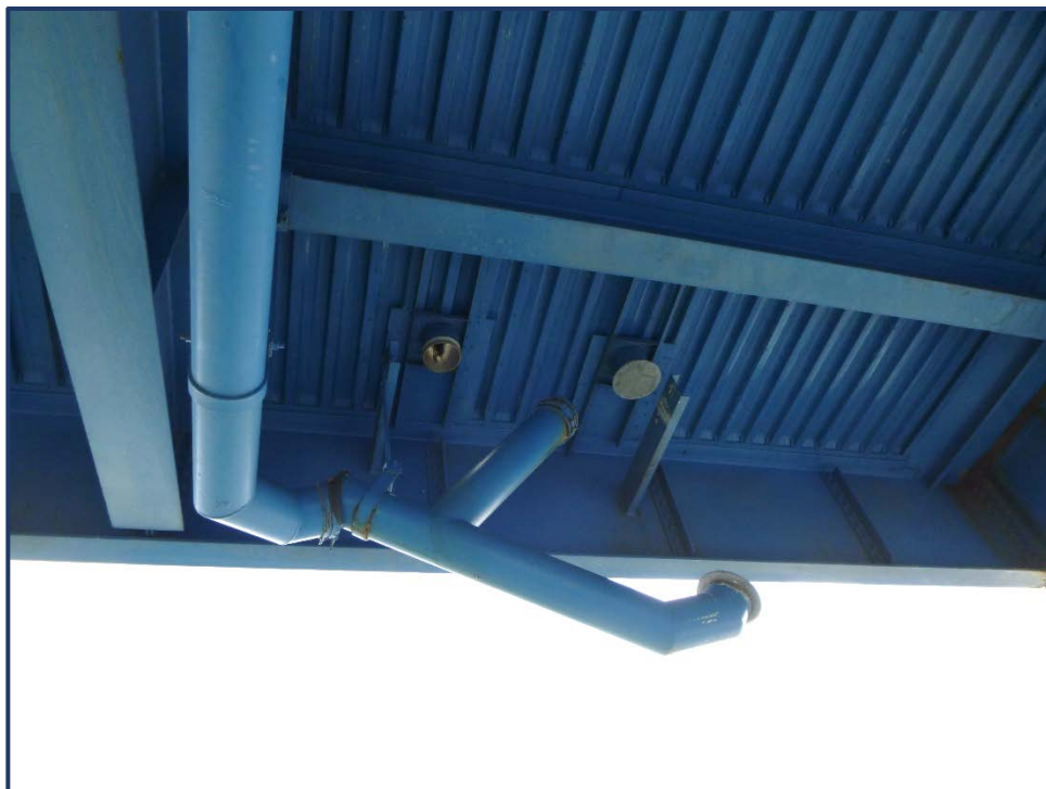
Photo 815-3 – Unit II, Span 9, North Side Scupper Downspout Disconnected
