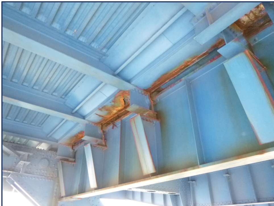
Photo 152-2 – Unit II, Span 8, FB 25, Active Surface Corrosion due to Deck Drainage
