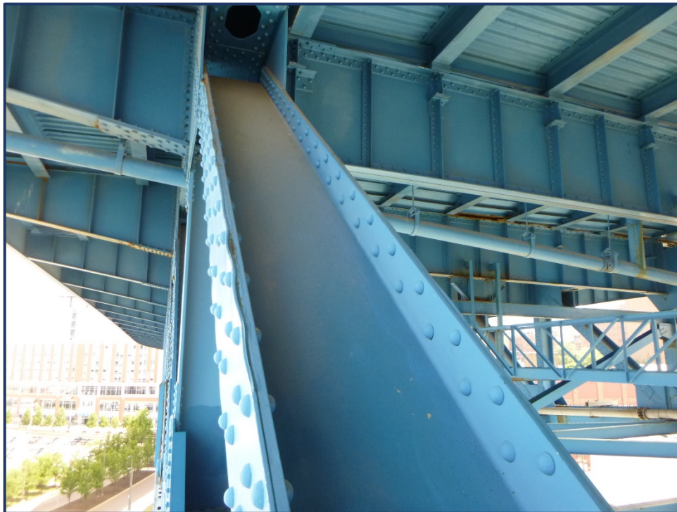
Photo 120-2 – Typical Distortion of Diagonal Flange Plates due to Sealed Pack Rust
