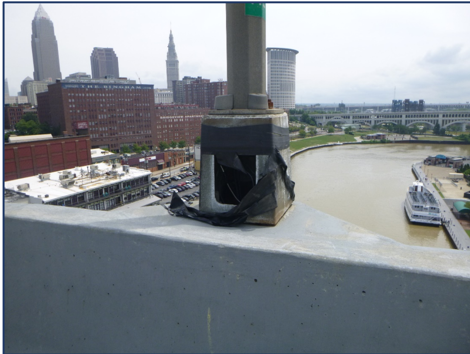
Photo LI-1 – Typical missing Utility Cover at Light Pole
