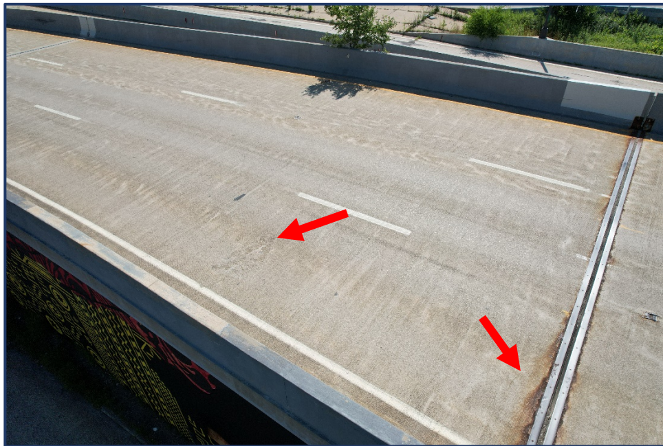
Photo 510-1 – Scaling of Wearing Surface and Shallow Spalls at Joint Header
