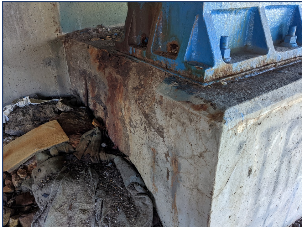
Photo 210-2 – Pier 37, Span 38 South Bearing Pedestal Spalling with Exposed Reinforcing
