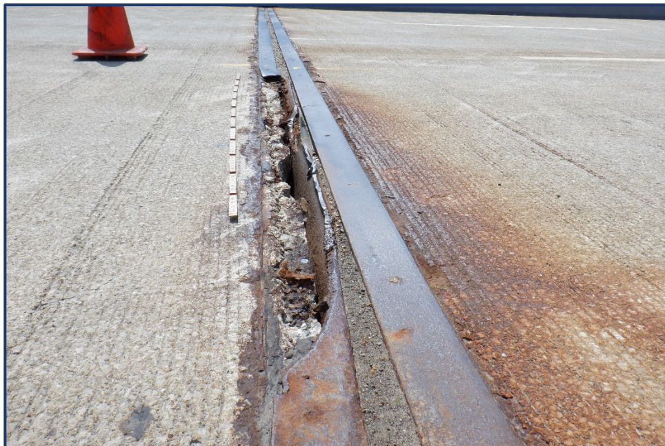
Photo 302-2 – Unit I, Joint X, 10-ft Section of Broken Retainer in Westbound Lane 3
