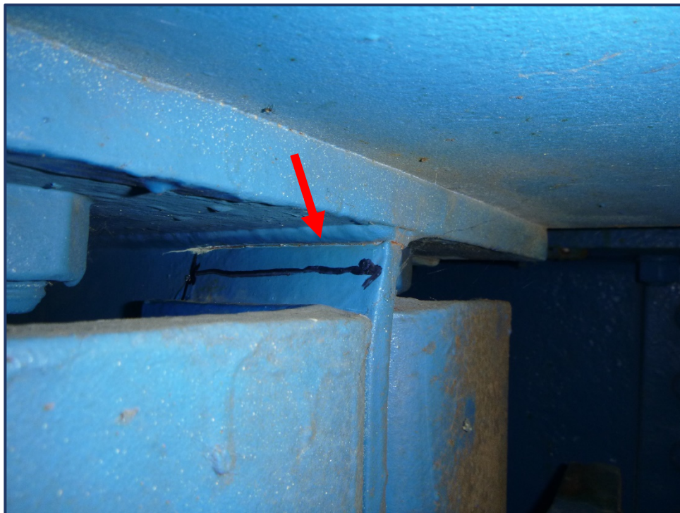
Photo 152-4 – Unit III, Span 11, FB 14 at North Truss, New Crack in OB Top Flange Cope
