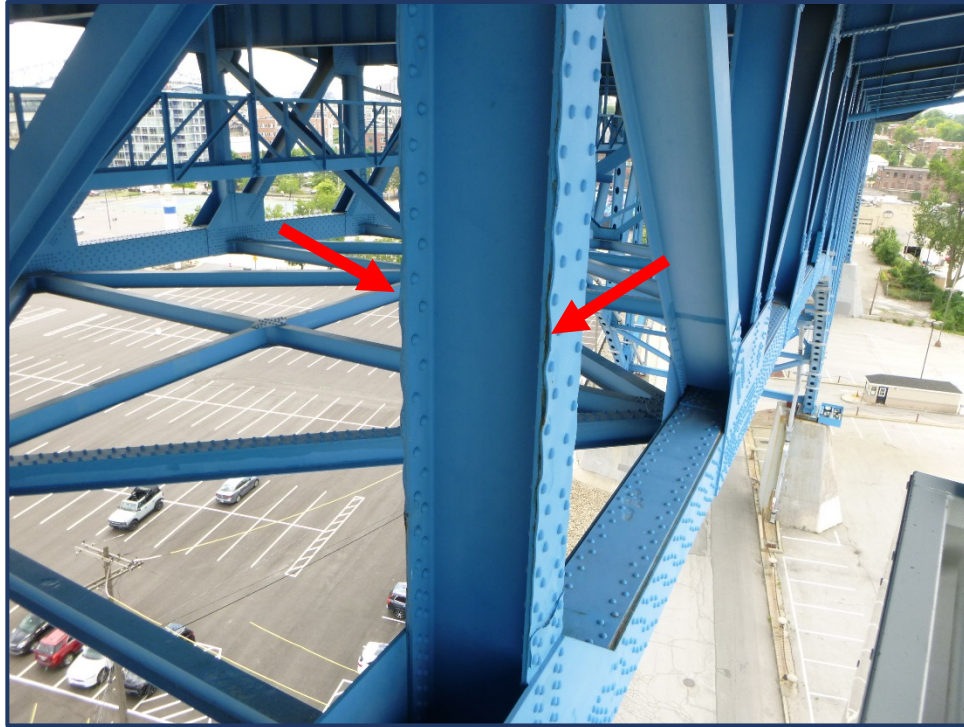
Photo 120-1 – Span 8, North Truss, L12-U12 Distortion of Cover Plates due to Pack Rust
