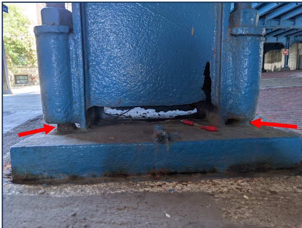
Photo 202-2 – Unit III, Bent 10 North Column, Painted Over Section Loss, Corrosion Holes, and Section Loss of Anchor Bolts
