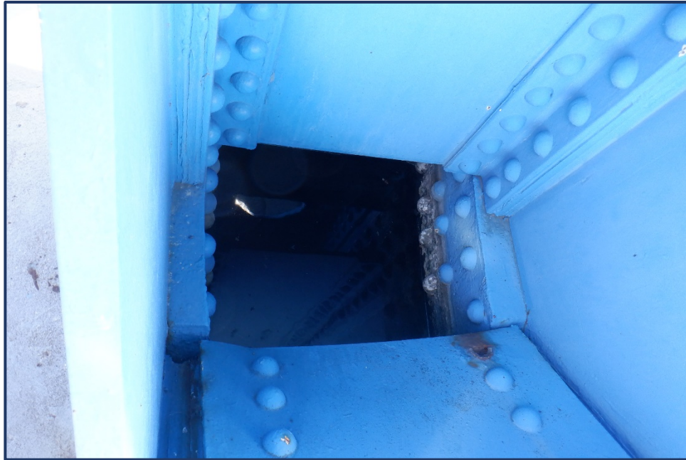
Photo 313-2 – Unit II, Pier 6, North Truss Bearing, Standing Water in Bearing
