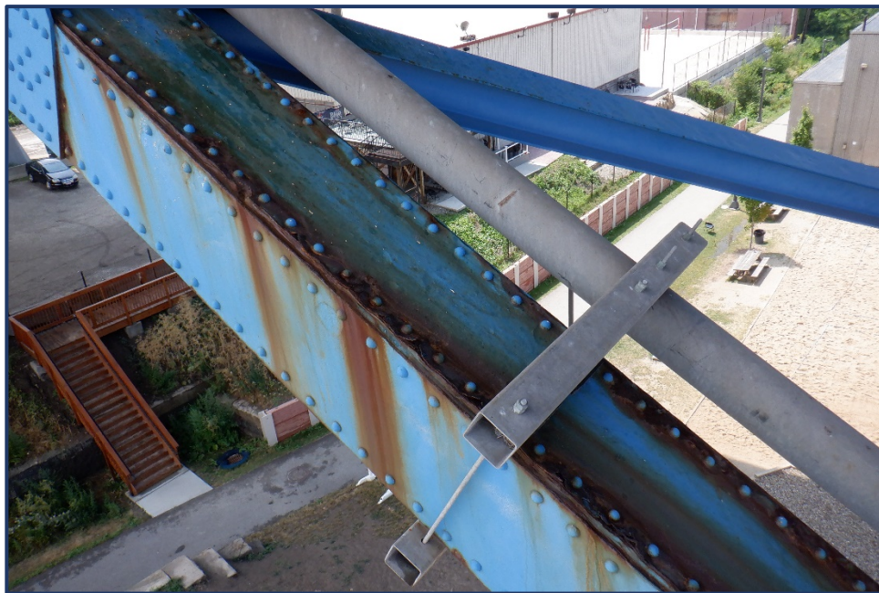
Photo 515-1 – Typical Active Corrosion near Deck Joint
