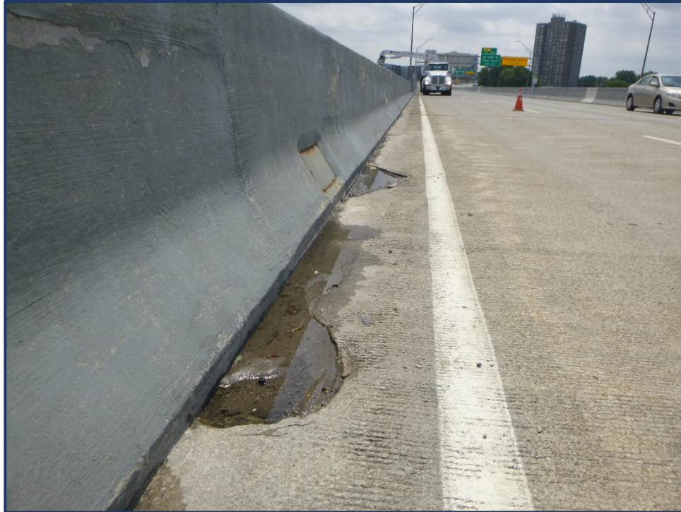
Photo 510-2 – Typical Spalling of Wearing Surface along Parapet
