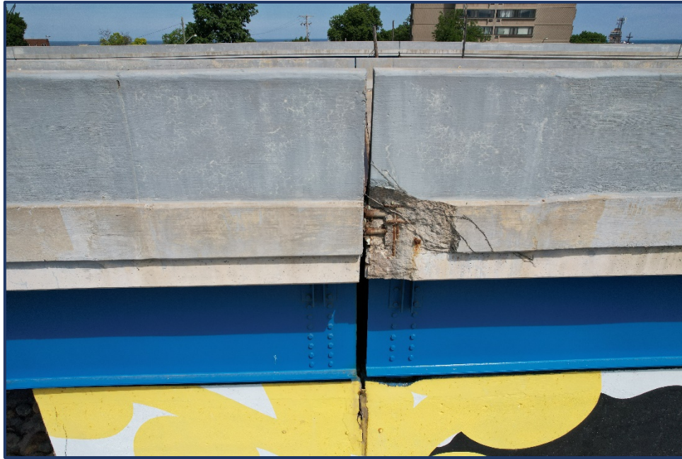
Photo 331-1 – Area of Parapet Spalling at Deck Joint.
