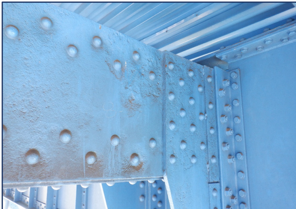
Photo 120-4 – Span 6, South Truss, U4-U5, Painted over Section Loss
