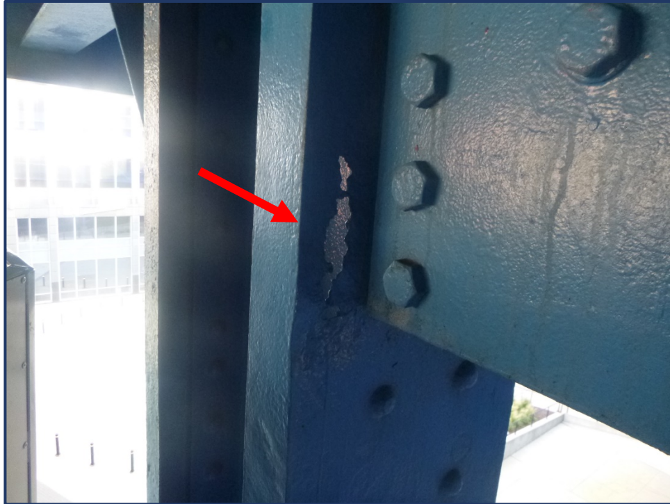
Photo 202-1 – Unit III, Bent 4 North Column, Painted Over Corrosion Hole at Bracing Connection
