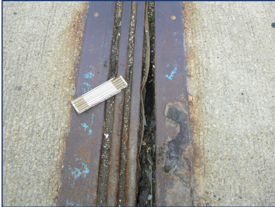
Photo 303-1 – Unit II, Joint K, Debris Impaction, Section Loss and Area of Tearing Joint Seal
