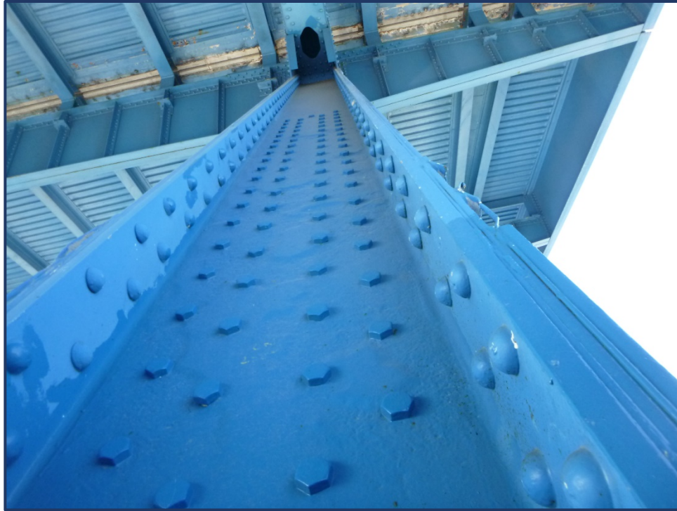
Photo 120-3 – Area of Painted over Section Loss on Diagonal with Retrofit Plate on Back Side
