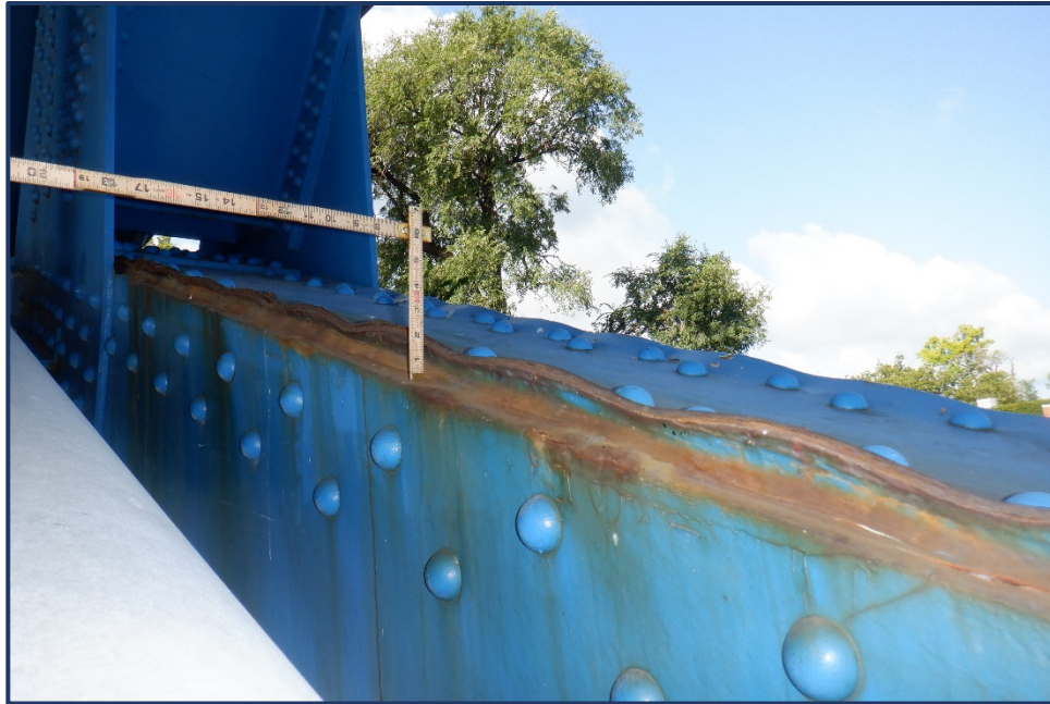
Photo 120-7 – Span 2, South Truss, L1-L2, Distortion of Top Flange Plate due to Pack Rust
