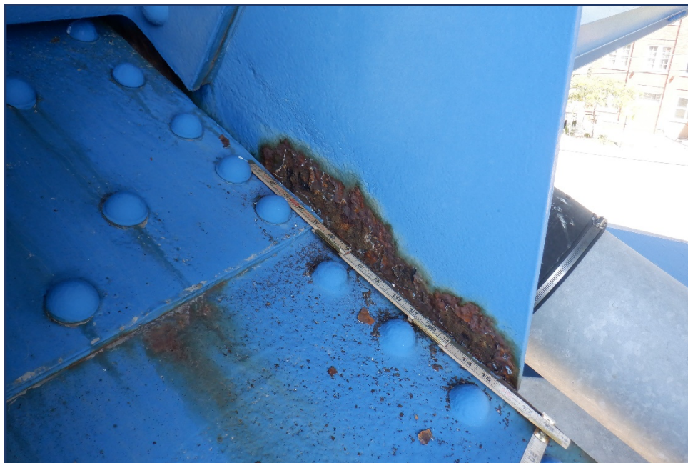
Photo 162-2 – Unit II, Span 2, South Truss, Reactivating Section Loss on L8 North Gusset Plate along Lower Chord
