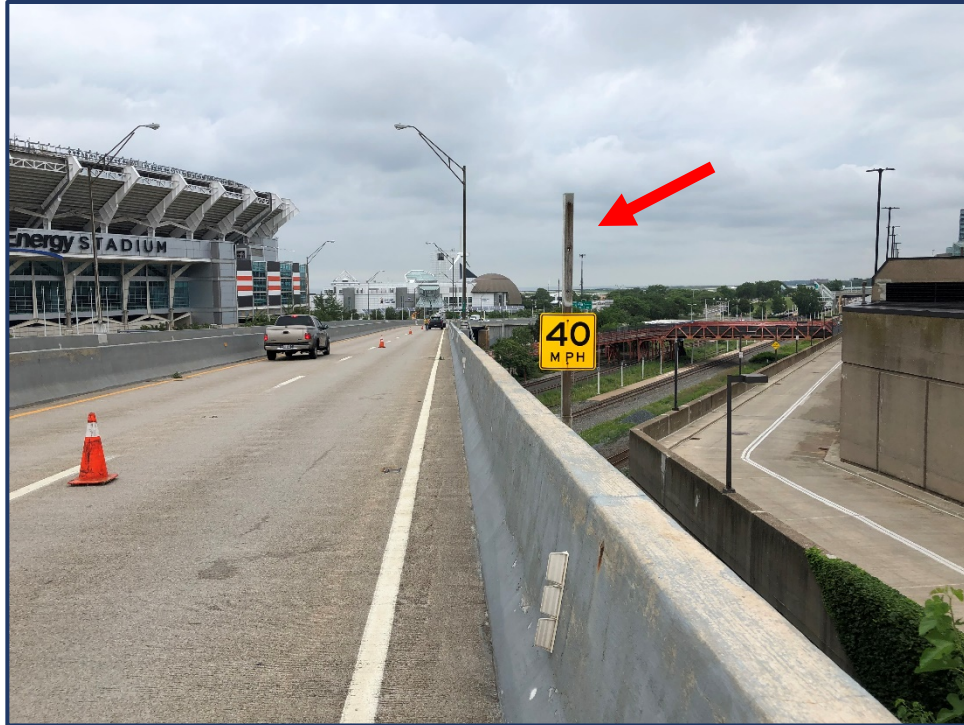
Photo SIG-1 – Unit V, Eastbound, Missing Sign on Right Parapet
