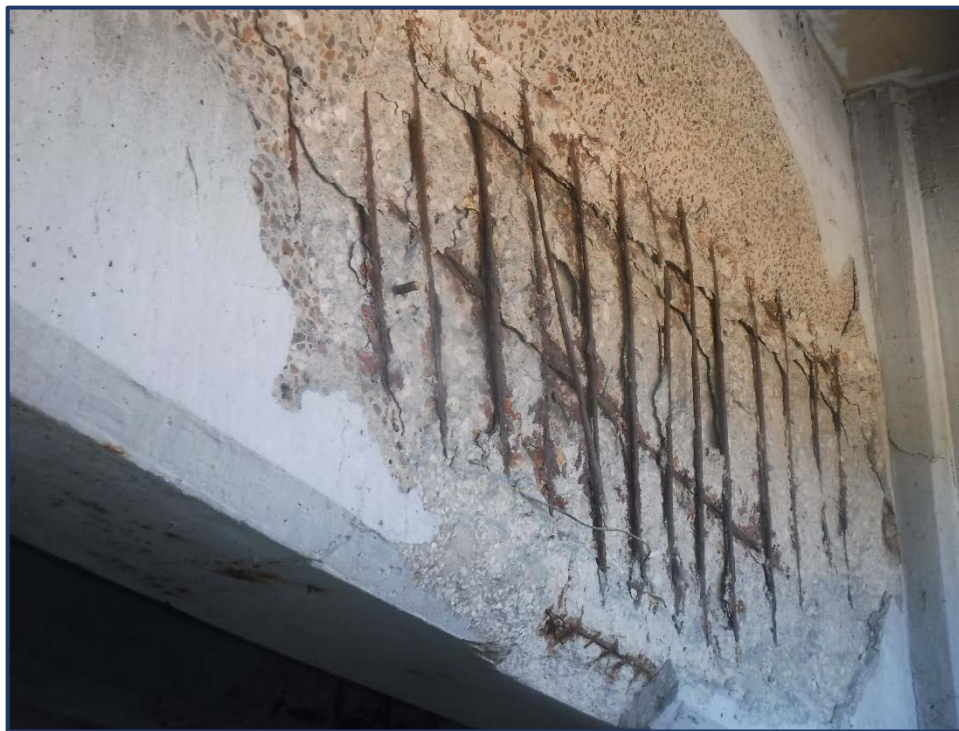
Photo 116-1 – Unit I, Section P, Girder 14, Spalling with Corroded Rebar
