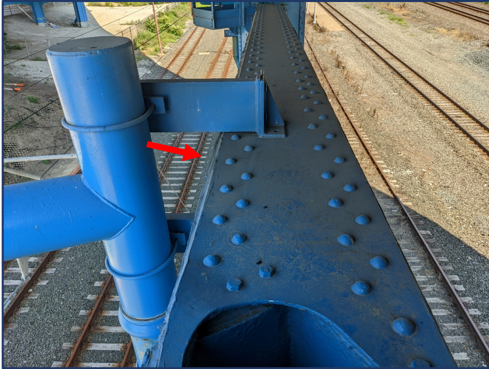
Photo 231-1 – Unit V, Pier 39, Painted over Pack Rust on Pier Cap
