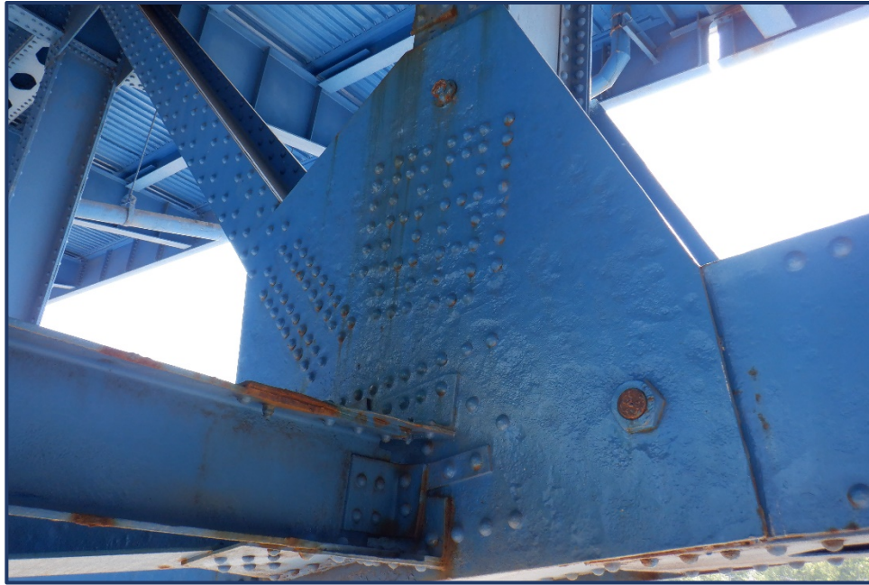
Photo 162-1 – Unit II, Span 1, South Truss, Painted Over Pitting on L7 Gusset Plate
