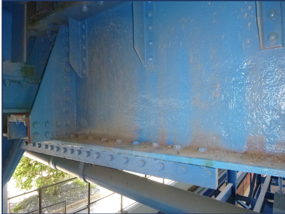
Photo 152-1 – Unit III, FB7, Painted over Section Loss in Lower Half of Floorbeam
