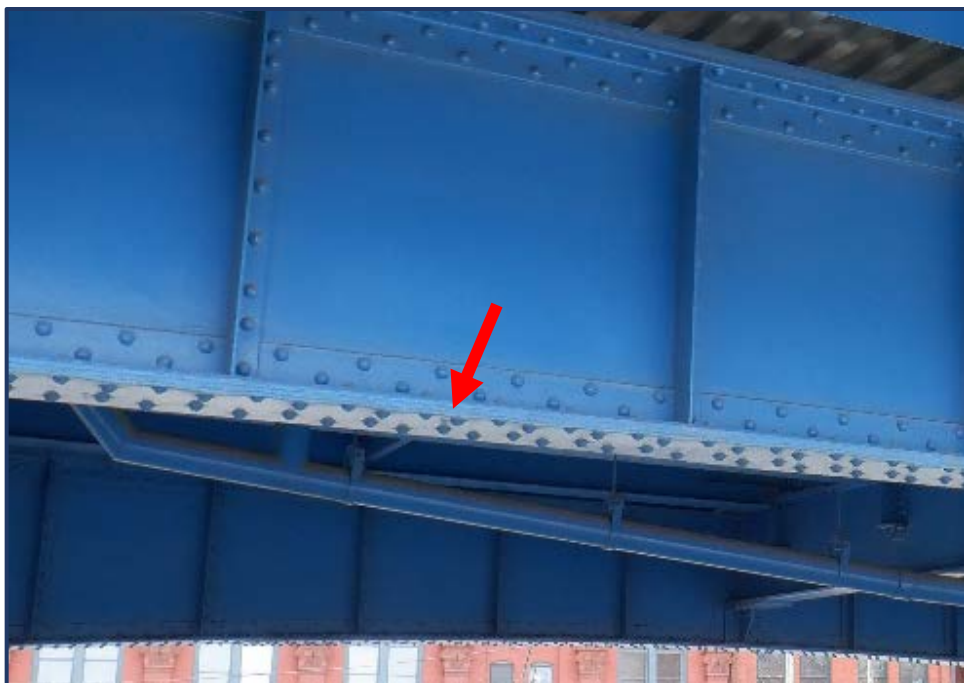
Photo 107-2 – Unit IV, North Girder at B22, Bottom Flange Painted over Pack Rust up to 1"
