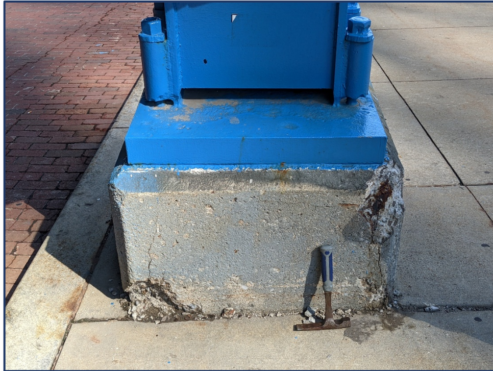
Photo 202-3 – Unit III, Bent 2 North Column, Cracking and Spalling of Column Base
