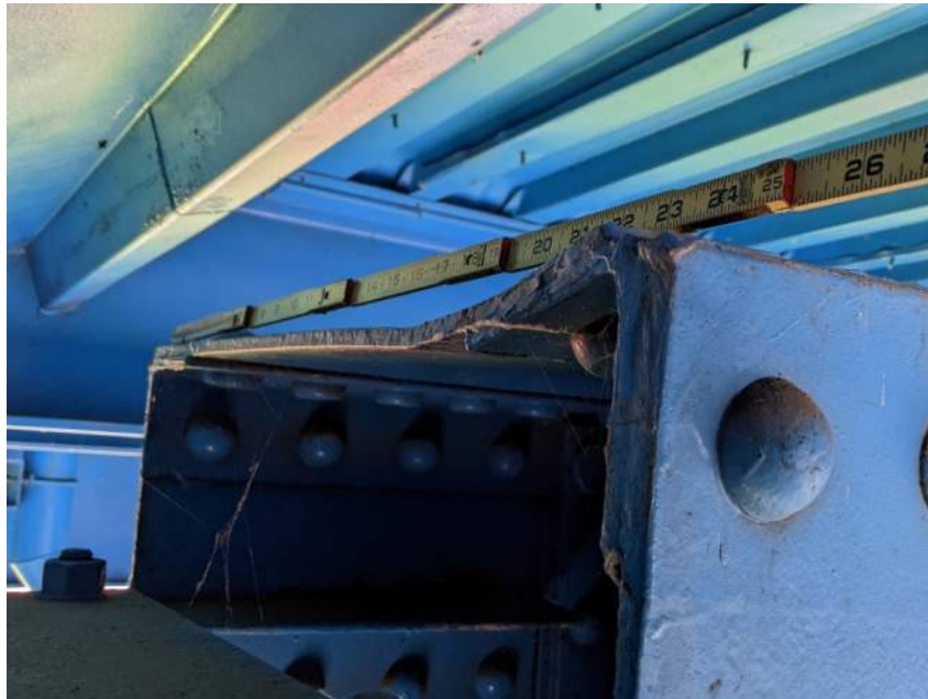
Photo 19: Bowing of Top Chord, Top Flange
