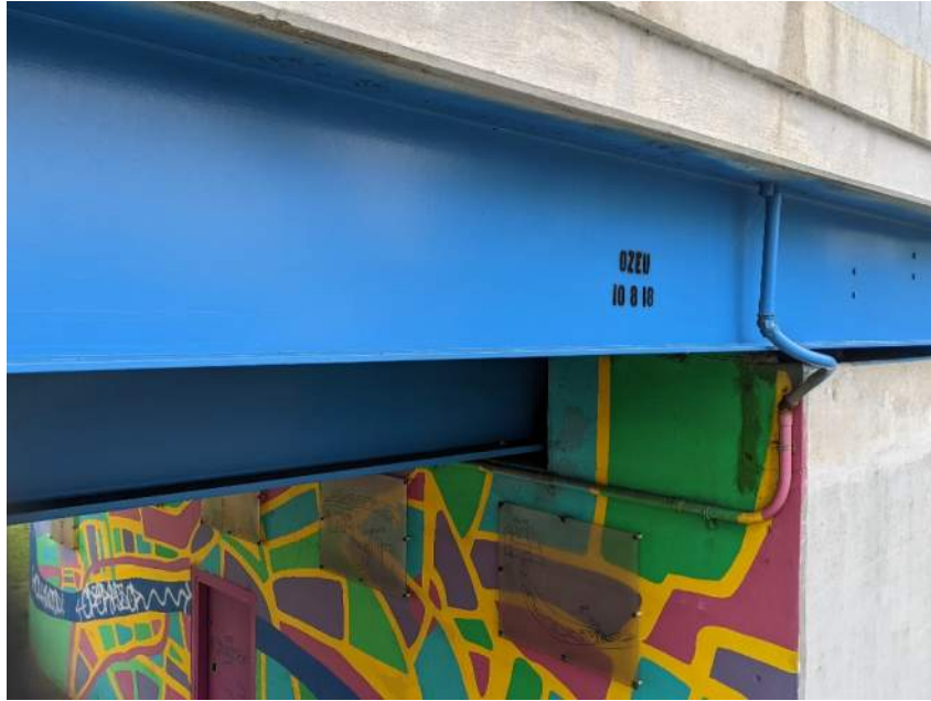
Photo 33: Protective Coating System in Unit I
