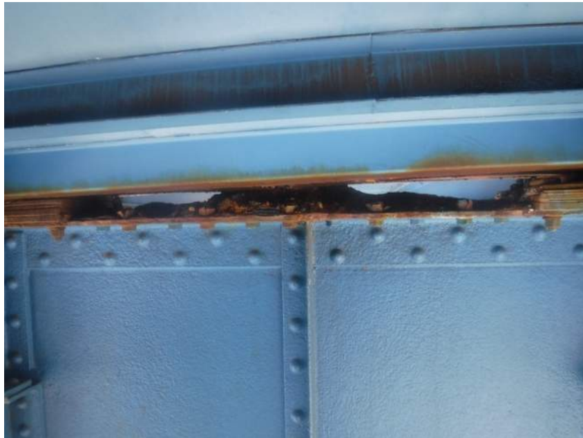
Photo 3: Visible Daylight and Debris Collection on Floorbeam Below Joint I1
