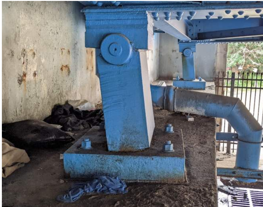
Photo 30: Painted Over Pitting of Movable Bearings at Abutment A
