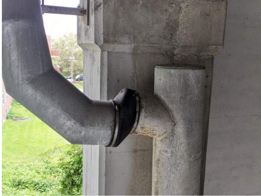
Photo 13: Misaligned Downspout in Unit I, Section P at North Fascia Near Joint O
