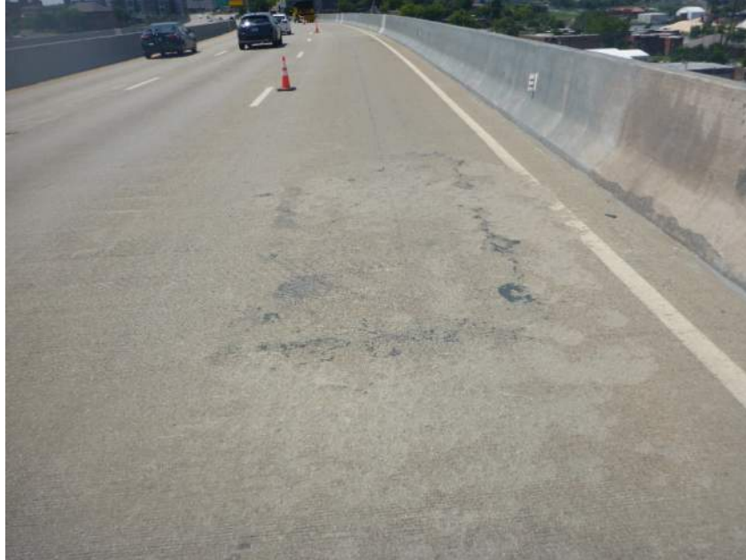
Photo 10: Wearing Surface Damage Due to Vehicle Fire in Right Westbound Lane In Unit II
