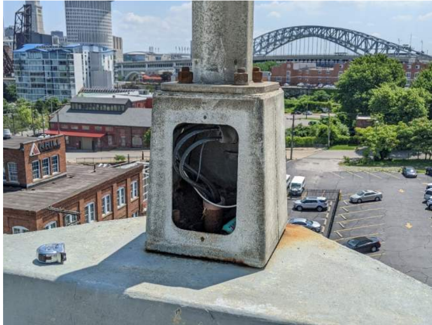
Photo 52: Missing Cover with Exposed Wiring At The Base Of A Light Pole
