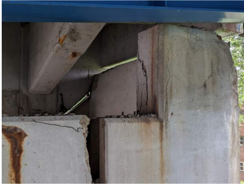
Photo 16: Reinforced Concrete Stringer with Cracking with Rust Staining Near North Fascia at End of Unit I at Joint O, Section P
