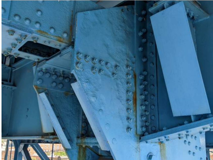
Photo 26: Painted over pitting at Span 6, U0, Outboard Gusset Plate
