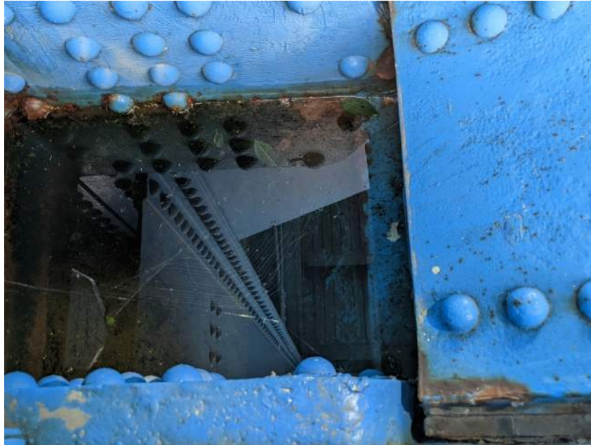
Photo 32: Standing Water in A Bearing Assembly in Unit II
