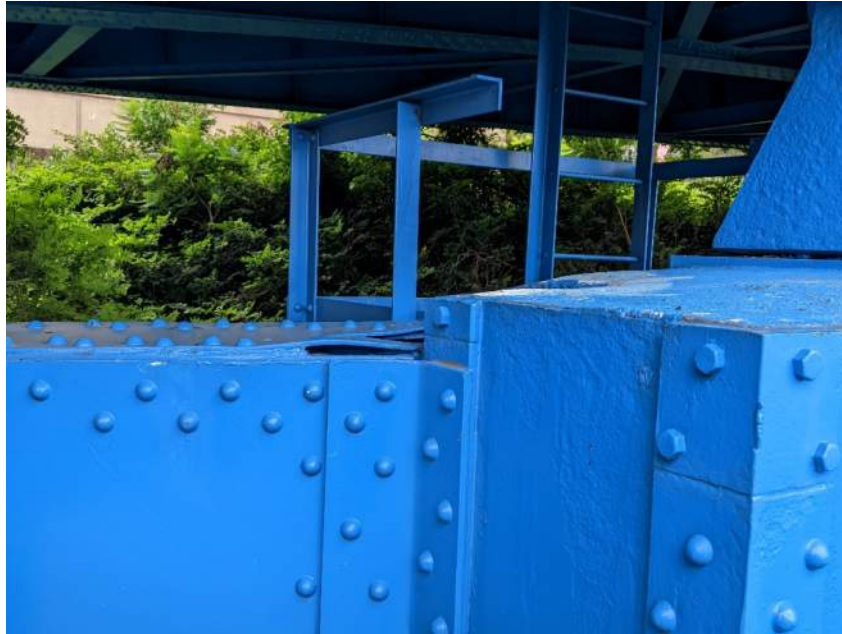
Photo 39: Unit V Steel Pier Cap Plate Distortion Due to Pack Rust
