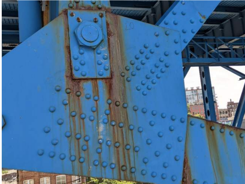
Photo 28: Rust Staining at Lower Chord Gusset Plate in Span 3 North Truss, L0
