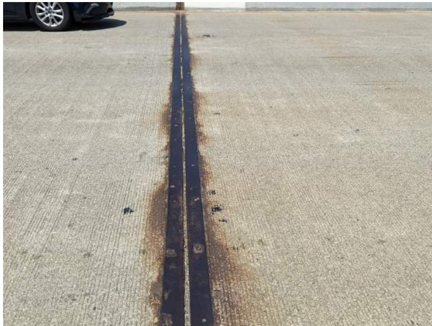
Photo 4: Typical Compression Seal Joint Debris Impaction
