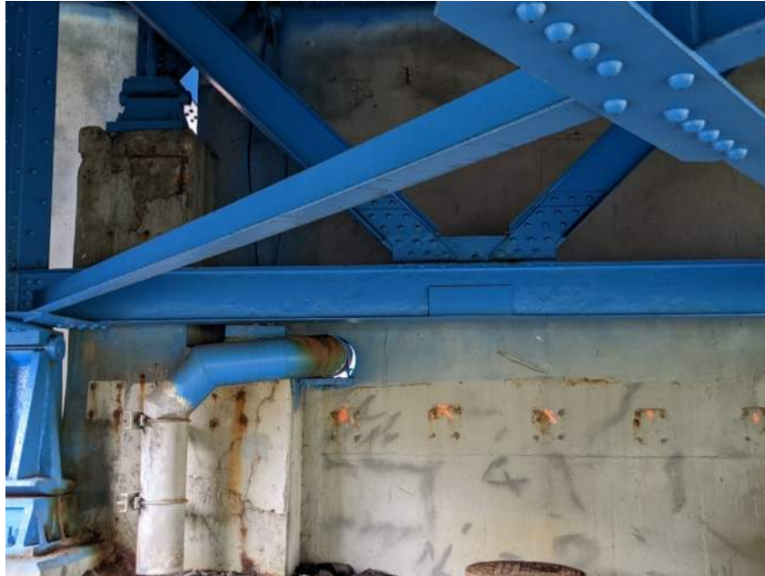
Photo 37: Pier 37 Bearing Pedestals Spalling
