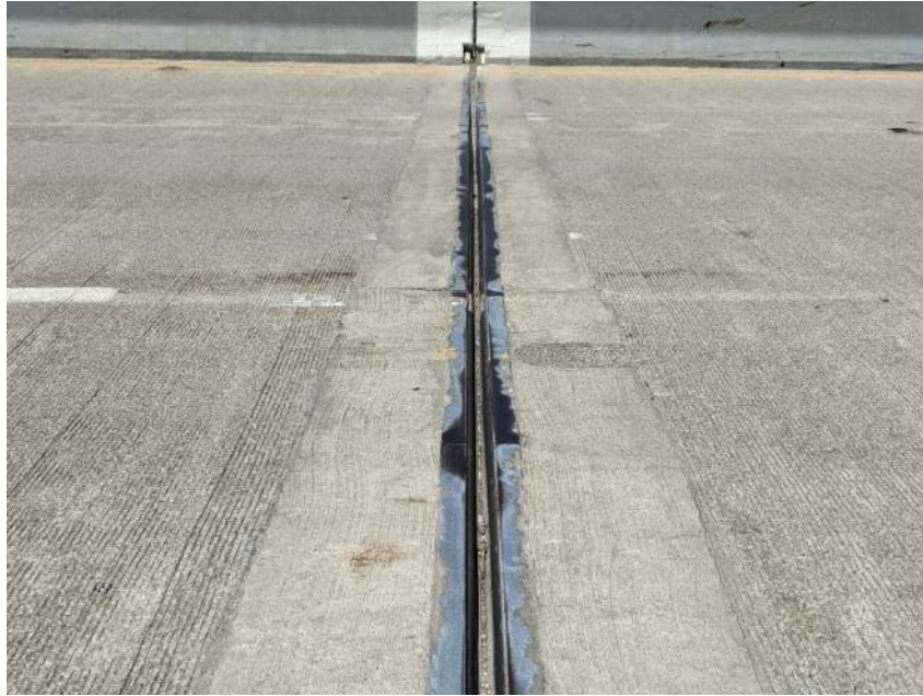
Photo 2: Typical Debris Impaction of Strip Seal Expansion Joints
