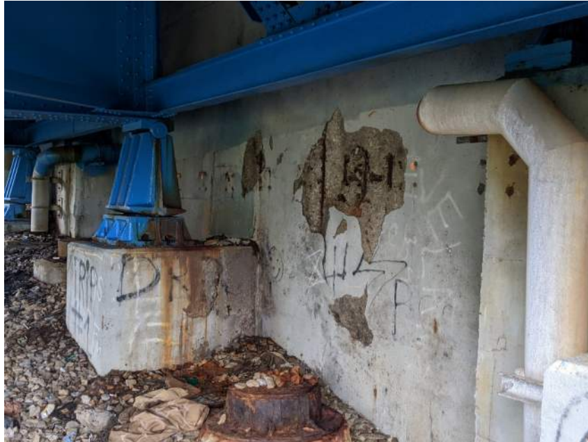
Photo 36: Pier 37 Wall Spalls
