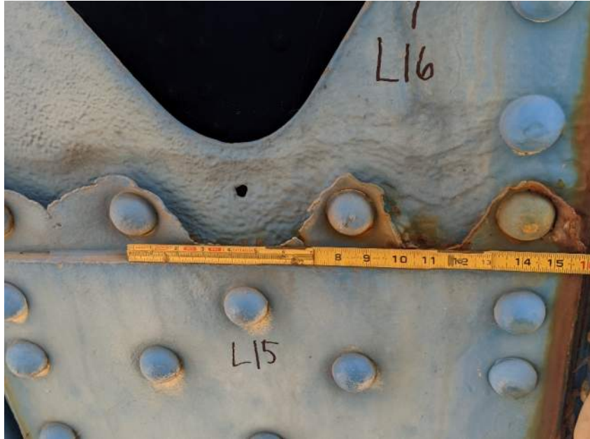
Photo 21: Painted Over Pitting, Pack Rust at Fill Plates of L15L16
