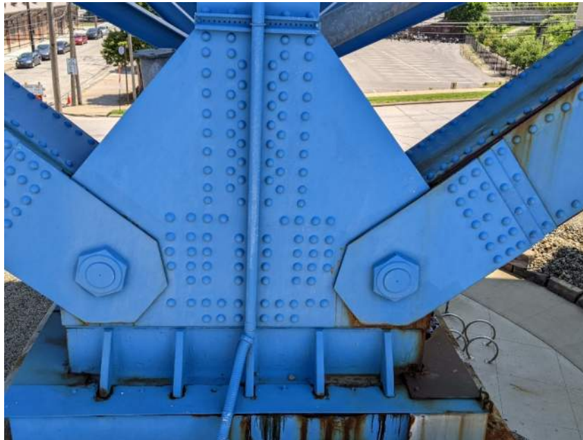
Photo 31: Typical Fixed Bearing with Moderate Corrosion
