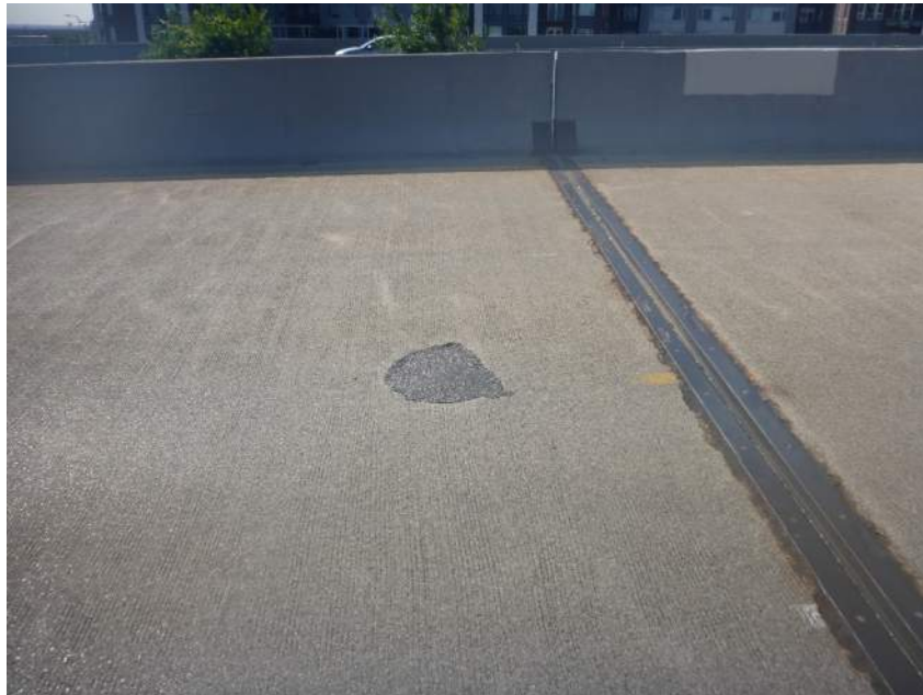
Photo 9: Wearing Surface Spall Patched with Asphalt
