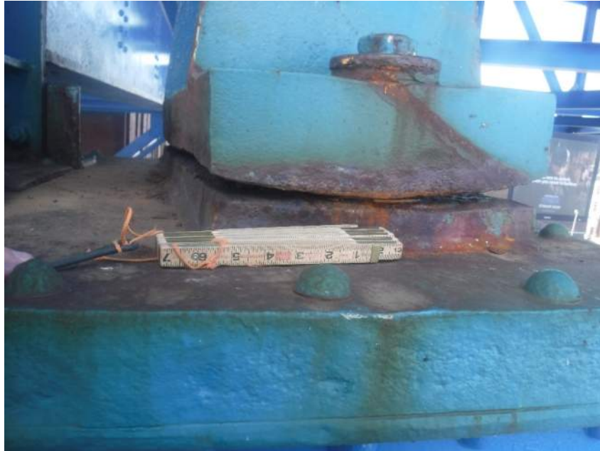
Photo 29: Active Corrosion with Section Loss Up To ¼" at Bearing Below L8 In Span 11
