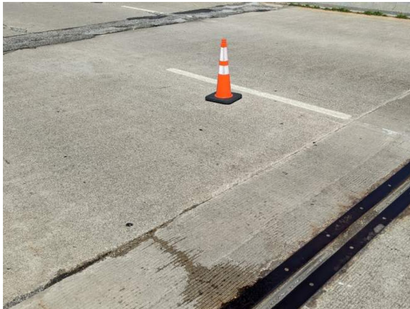
Photo 47: Approach Slab with Asphalt Patching At End Of Eastbound, West Approach
