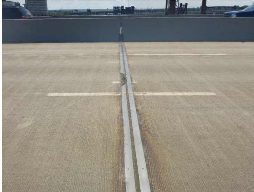
Photo 5: Missing Joint Armor on Eastbound Joint 8Q
