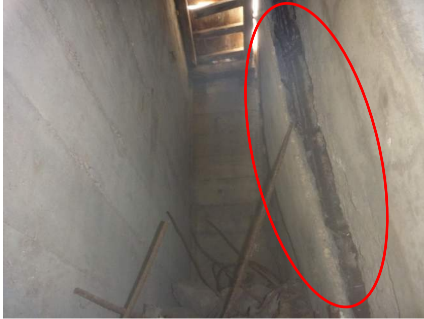
Photo 42: Section N Wall with Very Large Delamination
