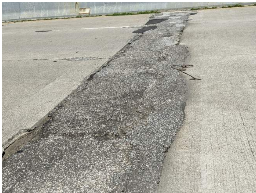
Photo 49: Asphalt Patching at End Of Eastbound, West Approach Slab
