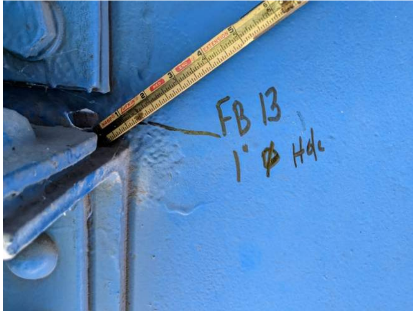
Photo 23: Painted Over Pitting and Corrosion Holes in Floorbeam
