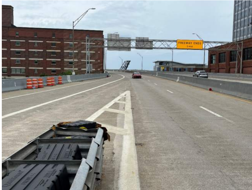
Photo 51: Damage to Impact Attenuator at Eastbound Exit to W. 6 th Street
