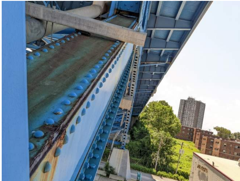
Photo 34: Protective Coating System with Reactivating Corrosion Near a Joint
