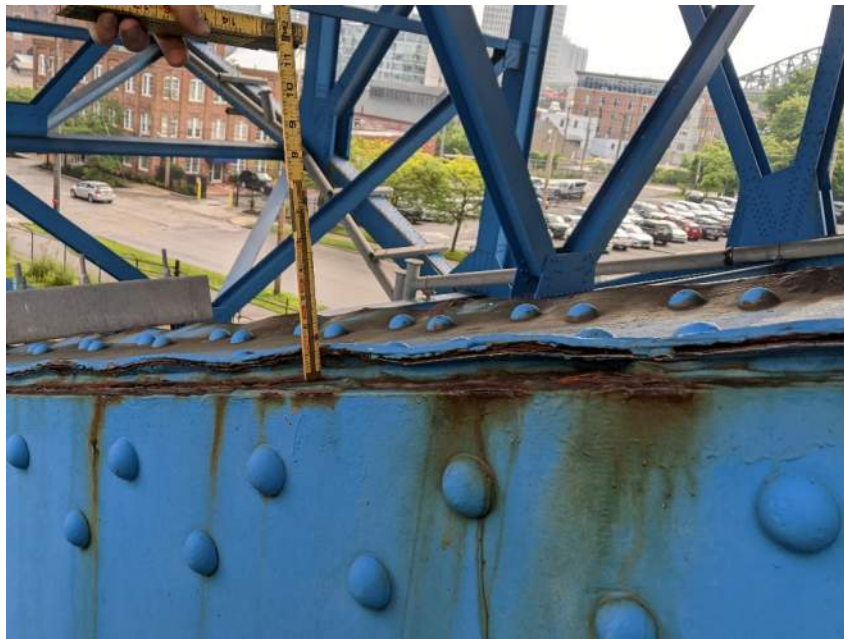
Photo 20: Painted Over and Reactivating Pack Rust Typical Between Web and Flange Plates
