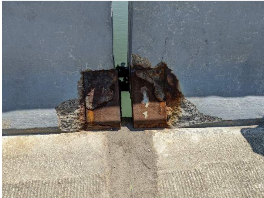
Photo 8: Typical Railing Spalls Adjacent to Joint Armor
