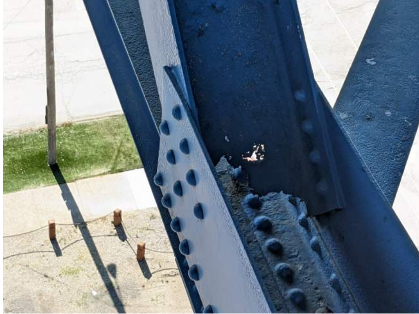
Photo 22: Painted Over Pitting and Corrosion Holes in Sway Bracing
