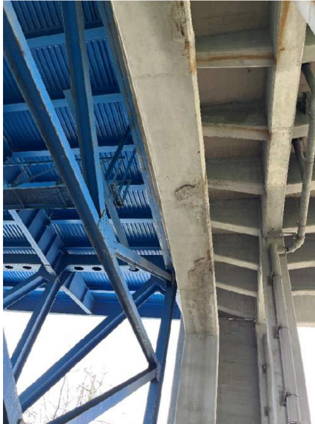
Photo 40: Underside of Pier O in Section P Delaminations
