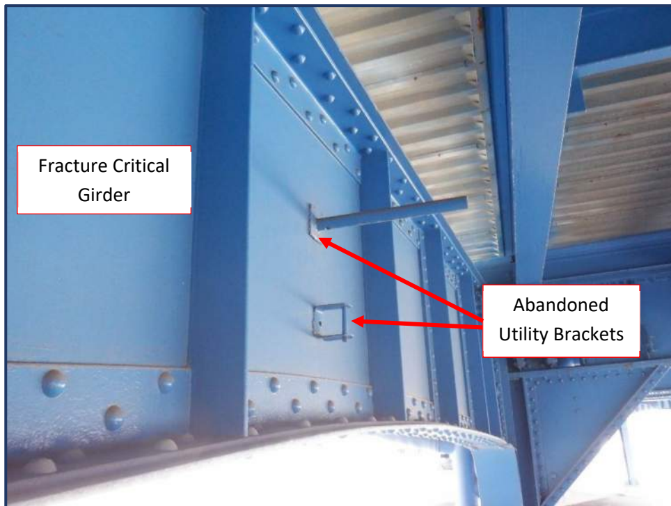
Photo 2 – Abandoned Utility Brackets on Unit IV Girder Webs
