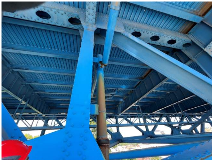
Photo 12: Disconnected Downspout in Unit II, Span 2, South Truss at U6L6
