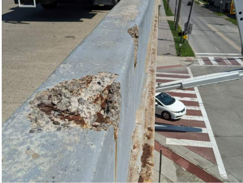
Photo 7: Railing spalls on South Railing, West of W. 25 th Street
