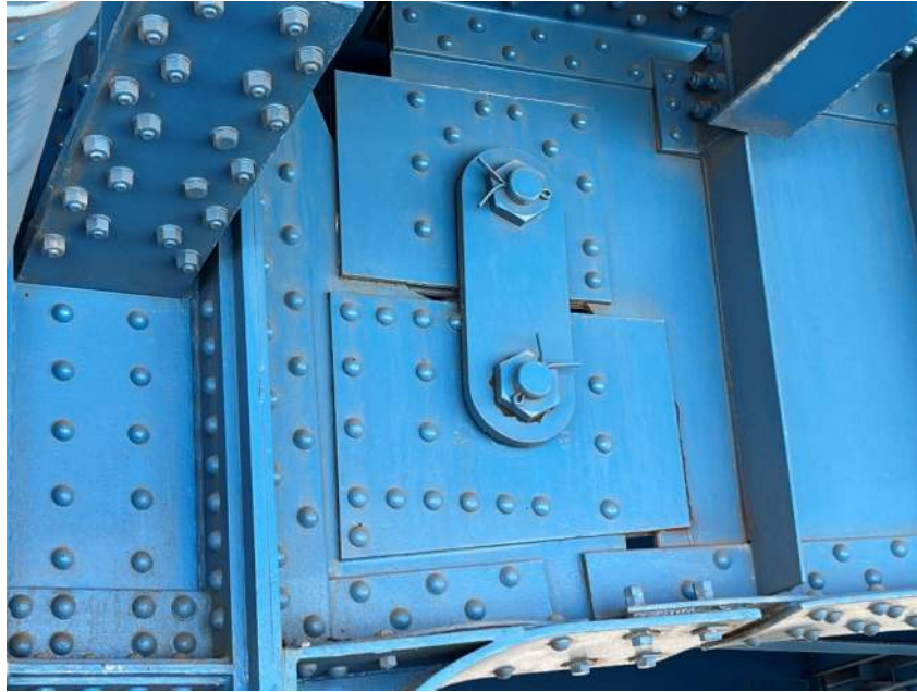
Photo 25: Pin and Hanger Assembly
