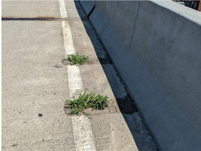
Photo 11: Typical Fully Clogged Scuppers
