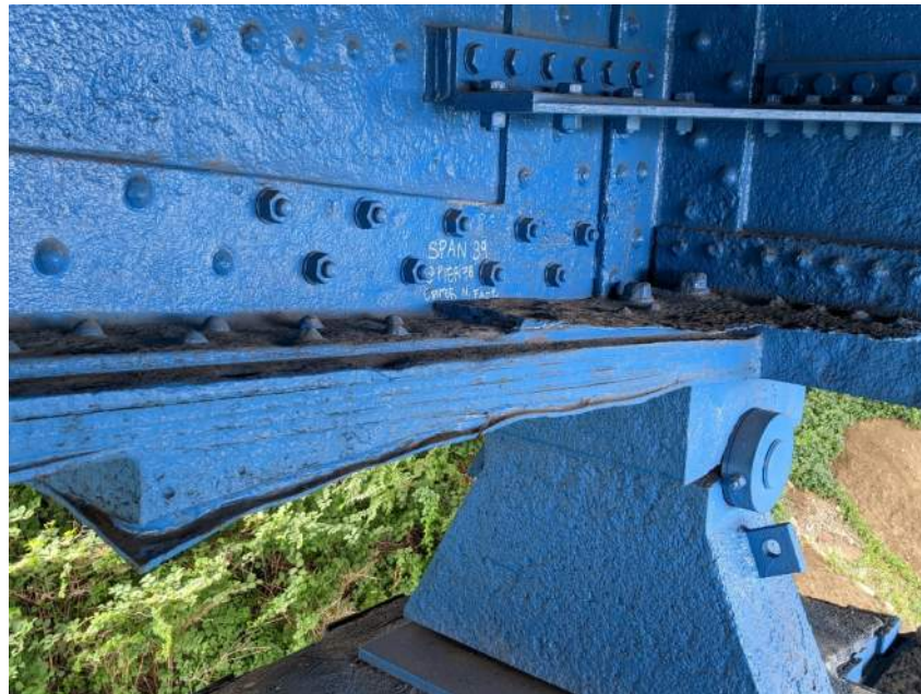
Photo 14: Pitting and Distorted Plates of Center Girder in Unit V, Span 39 at Pier 38, North Face
