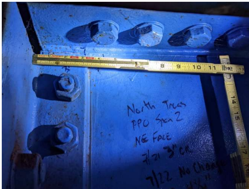
Photo 24: Propagating Crack in North Truss Floorbeam
