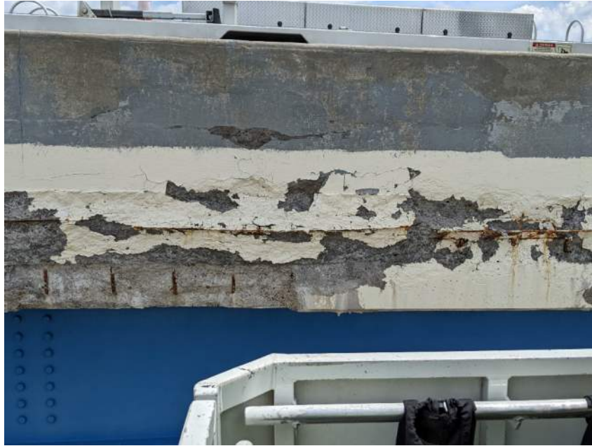
Photo 1: Deck Edge Spalling
