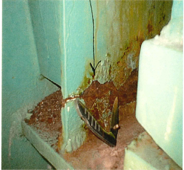
Picture 1- Initial Crack in the Upper Box Plate Photo/ODOT
