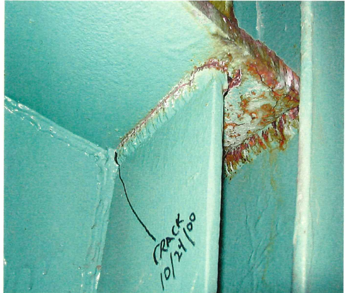
Picture 2 - Second Crack in Lower Box Plate Photo/ODOT
