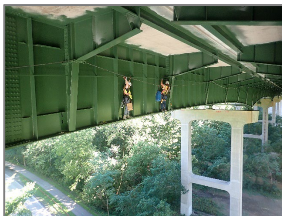
Photo 2 – Typical protected climbing and rope access techniques utilizing the safety cables along the girders, looking northeast at Girder D in Span 3.
