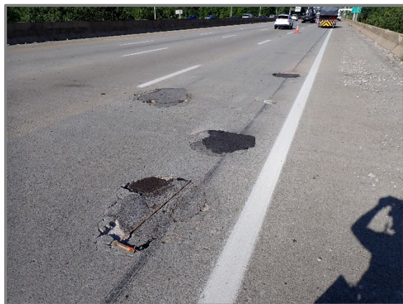
Photo 11 – Several potholes and failing patches in the right lane of the Span 6 wearing surface on the westbound structure, looking west.
