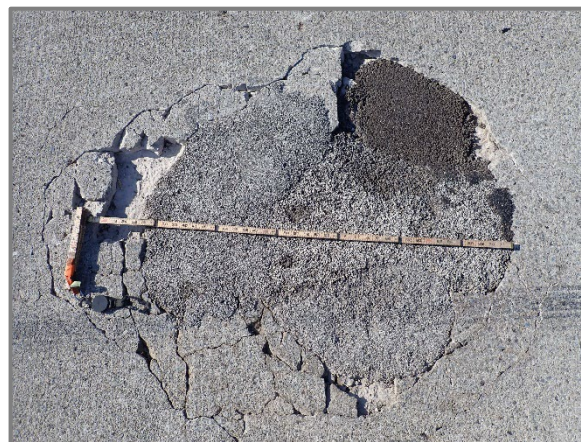
Photo 10 – Typical failing patch in the right lane of the westbound structure wearing surface in Span 5, looking south. Note additional broken up wearing surface material around the perimeter of the patch.
