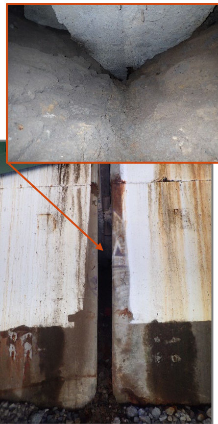
Photo 50 – Embankment fill spilling out from behind the Forward Abutment backwall through the median joint, looking north. Note the 8' tall by 15' wide by 30' deep void that has resulted below the approach slabs.
