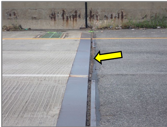
Photo 15 – Joint armor discontinuous and depressed approximately 1/2" at the westbound Rear Abutment joint in the 2 nd lane (from left).
