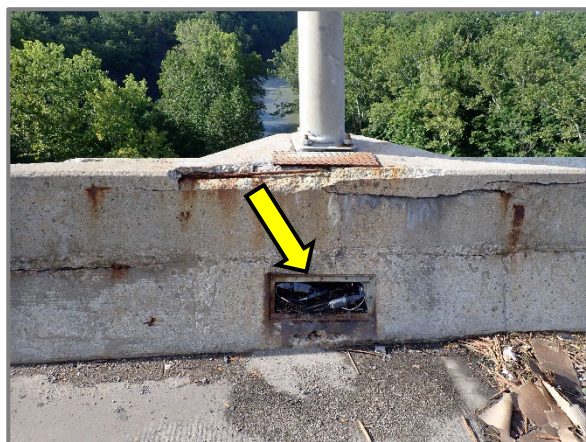
Photo 52 – Typical missing electrical panel access hatch below the light poles, looking north at Pier 7. Note exposed wiring, dirt, granular debris, and vegetation growth inside the panel.
