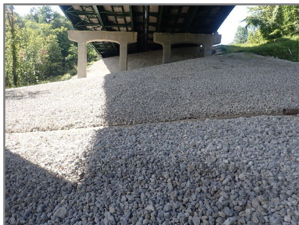
Photo 45 – Recently installed slope protection in front of the Rear Abutment, looking west.
