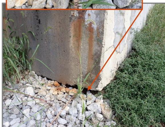
Photo 42 – Forward Abutment backwall and wingwall for the eastbound structure undermined up to 30" deep/long at its south end, looking east.
