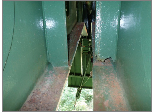
Photo 31– South cantilever of Floorbeam 26 on the westbound structure with 100% section loss at the base of a transverse stiffener near the base, looking south.
