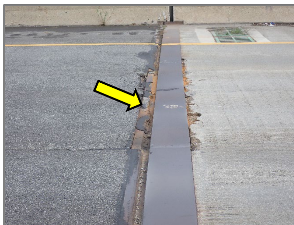
Photo 14 – 1/2" vertical misalignment at the Rear Abutment joint for the eastbound structure, looking north. Note the adjacent spalling to the joint header and that this joint bounces under live load traffic in the 2 nd lane (from left).
