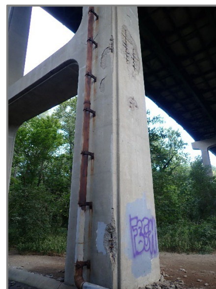
Photo 37 – Numerous delaminations and spalls with exposed reinforcement throughout the north column at Pier 3 of the eastbound structure, looking southwest.
