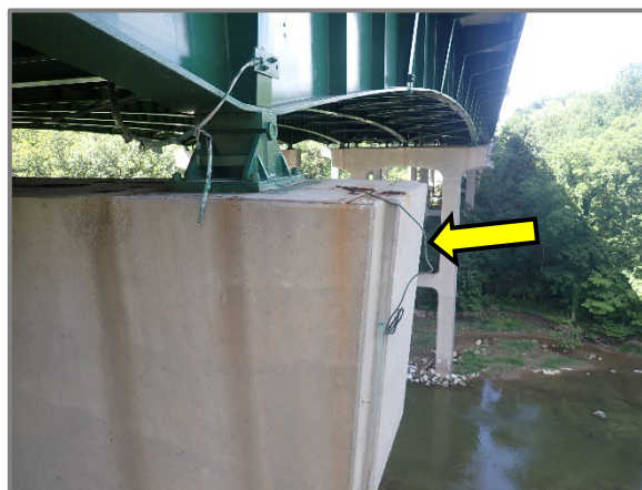
Photo 53 – Typical broken grounding cable at the pier caps, looking west at Pier 7 adjacent to Girder F.
