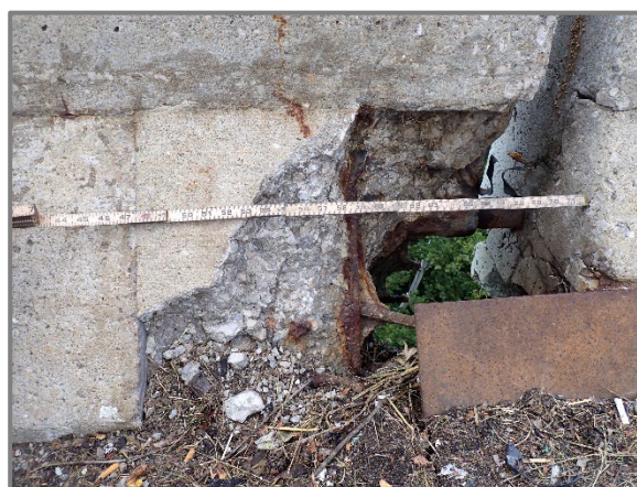
Photo 19 – 24" long by 24" high by full depth spall in the south bridge railing on the east side of the Span 6 joint on the eastbound structure, looking south. Note that spalls of this nature are typically present at the hinge joints.
