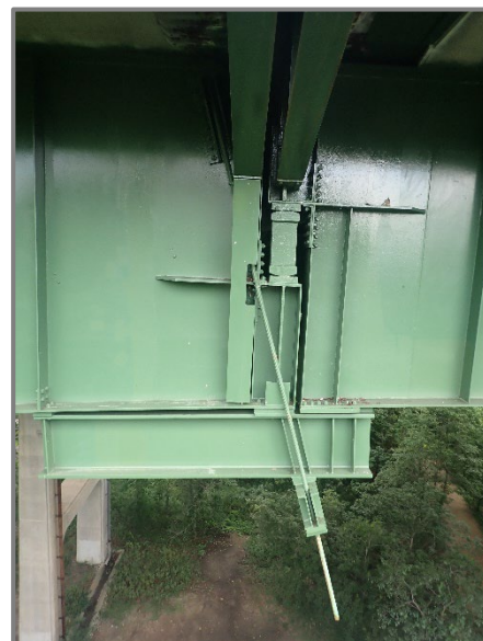
Photo 35 – Typical carrier beam retrofit installed below the seated hinge joints, looking north at Girder A at the Span 4 expansion joint.
