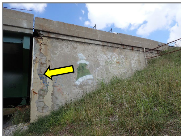
Photo 43 – 12" wide patch beginning to fail in the south wingwall at the along the Forward Abutment connection, looking north.
