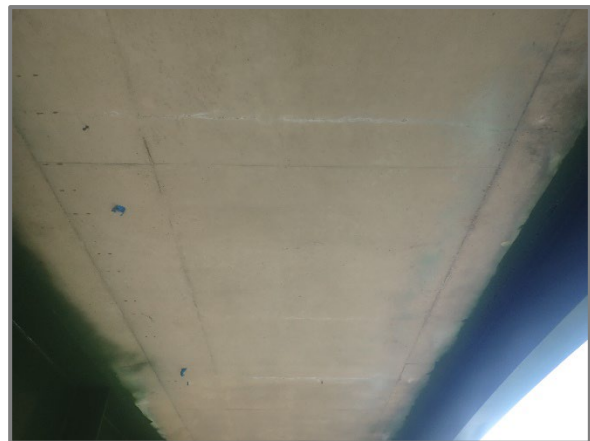
Photo 5 – Typical hairline transverse cracks with light efflorescence in the deck overhangs, looking east at the south overhang of the eastbound structure between Floorbeams 10 and 11, looking east.
