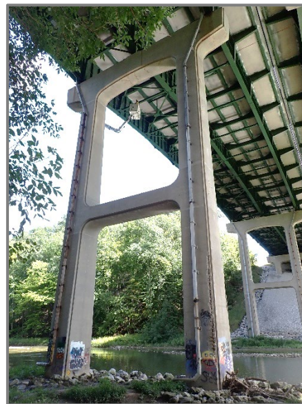
Photo 23 – West elevation of Pier 5 of the westbound structure, looking northeast. Note minor to moderate corrosion of the downspouts and large rubble rip rap in place at the column bases.
