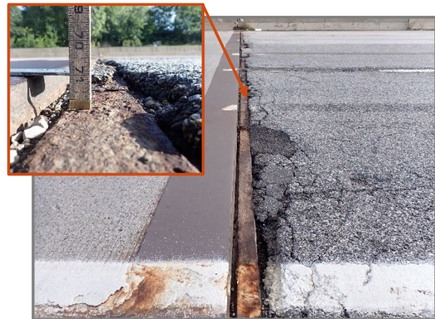
Photo 16 – Up to 1" vertical misalignment at the eastbound Forward Abutment joint in the right two lanes, looking north. Note the broken up joint header on the approach side with previous patches beginning to fail.
