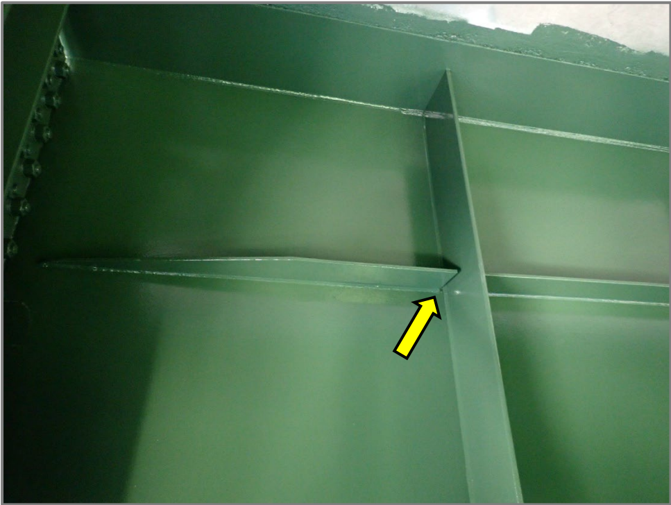
Photo 1 – Base metal at the end termination of longitudinal stiffener to girder web welds with no transition radius (Category E). Girder E at Floorbeam 18 shown, looking northeast.
