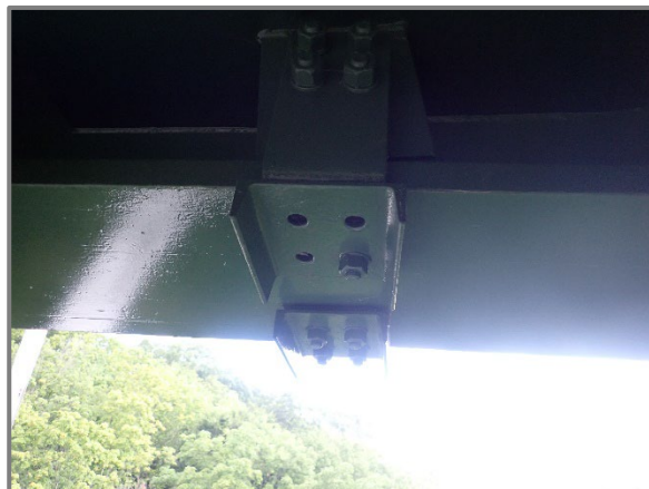
Photo 28 – 3 of 4 bottom flange bolts missing in the Girder F knee brace connection retrofit at Floorbeam 15, looking north.
