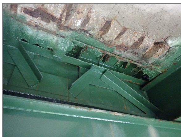
Photo 7 – 7' wide by up to 15" long by full depth spall with two layers of fully exposed and corroded reinforcement at the end of the eastbound structure deck along the Span 6 expansion joint armor, looking east.
