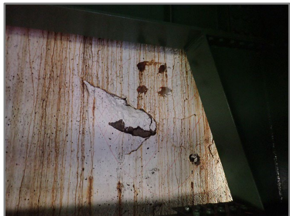
Photo 41 – 8' wide by 4' delamination with an adjacent spall in the Rear Abutment backwall behind Girder F, looking west.
