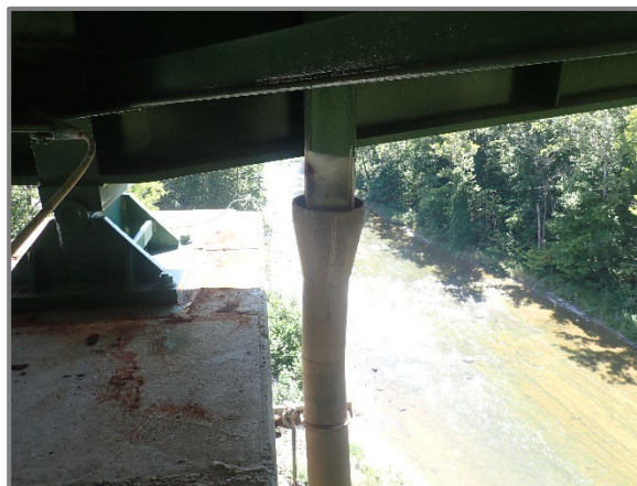
Photo 25 – Downspout at Pier 7 for the eastbound bridge fully clogged approximately 12' from the top, looking south.
