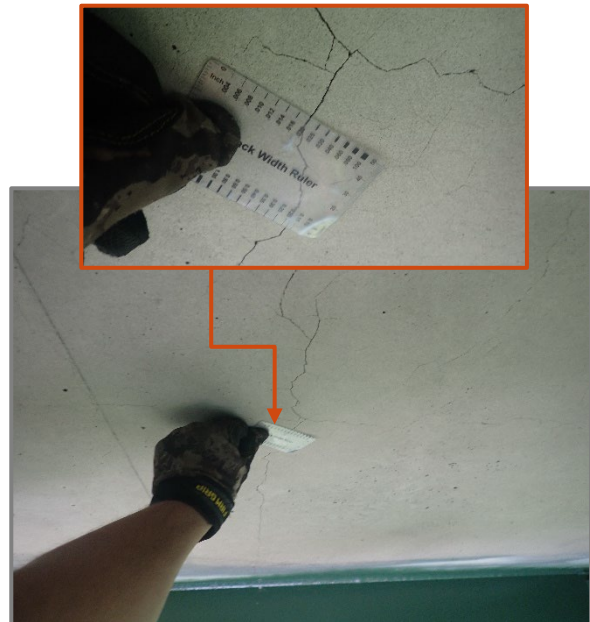
Photo 3 – 0.020" wide transverse crack in the Span 4 underside of deck between Floorbeams 24 and 25 of the eastbound structure, looking south.
