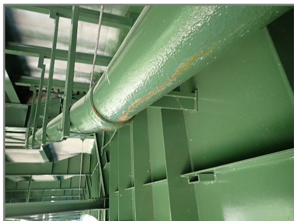
Photo 24 – Evidence of leakage in the north downspout near the hinge joint in Span 6 of the westbound structure, looking west. Note that corrosion holes were observed during the 2020 inspection but have not been noted since.
