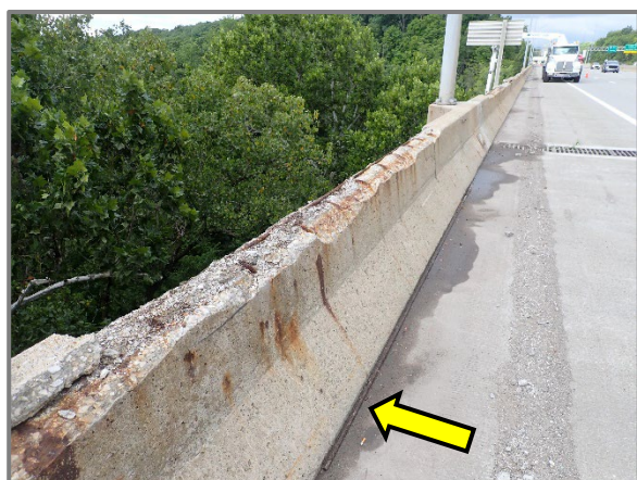
Photo 18 – Typical full width spalls with exposed, corroded, missing, and debonded reinforcement along the top edges of the exterior bridge railings, looking west at the south railing in Span 5 of the eastbound structure. Note the missing bar laying at the base of the railing.
