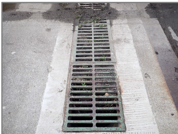
Photo 21 – Typical partially clogged drainage scupper (approximately 85% clogged), looking south at the west end of the bridge on the eastbound structure.
