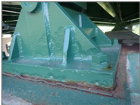
Photo 33 – Up to 1/4" deep cleaned and painted pitting on the bearing assembly and masonry plate for Girder F at Pier 7, looking south.
