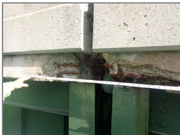
Photo 9 – Large spalls with multiple layers of exposed and corroded reinforcement in the south deck edge of the eastbound structure at the Span 4 expansion joint, looking northwest.
