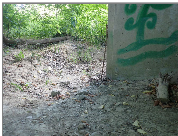
Photo 39 – Minor localized scour along the base of Pier 5 columns, looking south at the south column on the westbound structure.
