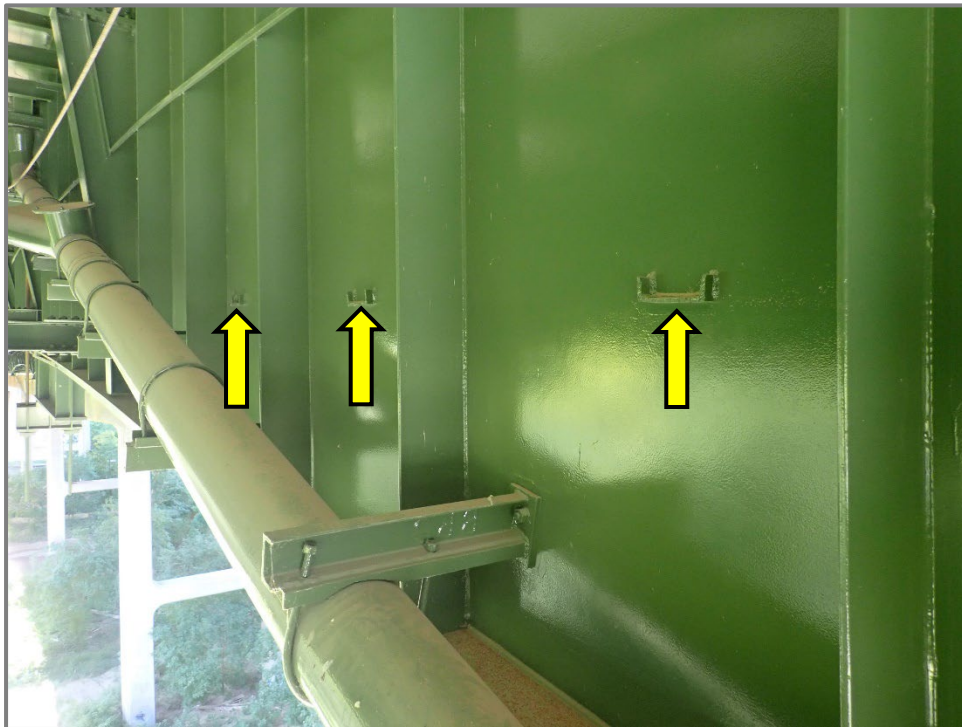
Photo 3 – Base metal at abandoned channel bracket to girder web welds (Category E). Girder C between Floorbeams 52 and 53 shown, looking northwest.
