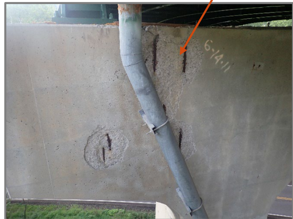
Photo 40 – 72" high by 42" wide by 2" deep spall with exposed and corroded reinforcement behind the downspout on the west face of the Pier 2 cap for the westbound structure, looking east.
