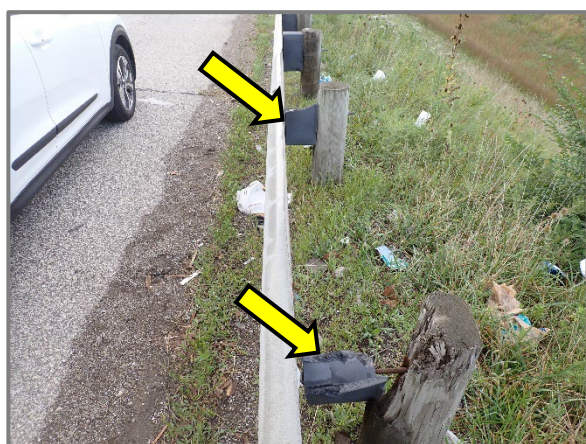
Photo 51 – Damaged timber posts and plastic blockouts on Posts 3 through 6 from the bridge end in the southeast corner approach guardfence, looking east.
