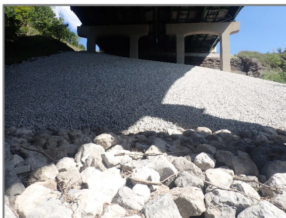
Photo 46 – Recently installed slope protection in front of the Forward Abutment, looking east.
