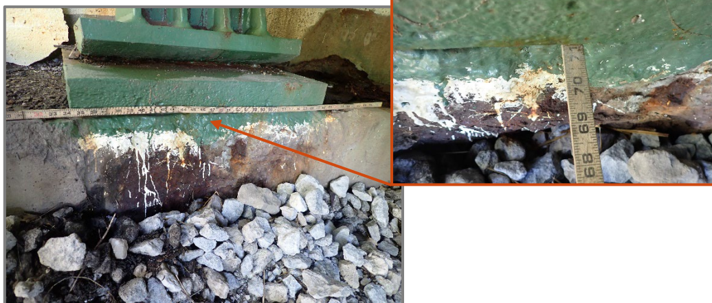
Photo 32 – Spall in the west face of the Girder F seat pedestal at the Forward Abutment undermining the bearing masonry plate up to 3/4" deep, looking east.
