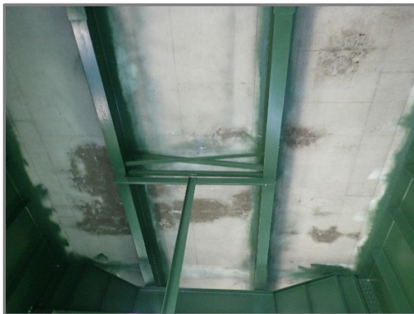
Photo 4 – Several areas of moisture staining and efflorescence in the deck underside between Girders E and F between Floorbeams 43 and 44, looking west. Note these locations are defects are typically located between failing patches in the wearing surface.
