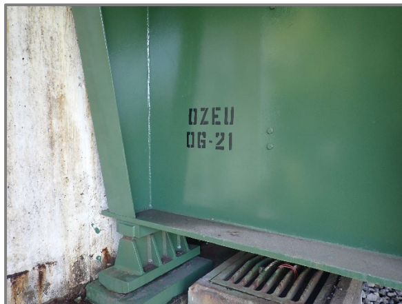
Photo 34 – New stamp denoting the recently applied OZEU protective coating system, looking northwest at Girder A at the Rear Abutment.
