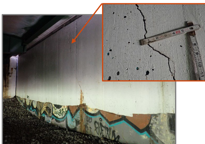
Photo 44 – 1/8" wide vertical/diagonal crack with moderate efflorescence and light rust staining in the interior wingwall at the Rear Abutment, looking northwest.
