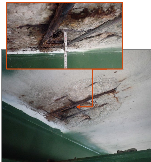
Photo 6 – 36" long by 42" wide by 5" deep spall with debonded and corroded reinforcement along the south side of Stringer 11 at Floorbeam 42 on the westbound structure, looking northeast.
