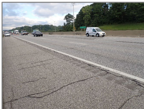
Photo 49 – Typical transverse and longitudinal cracks in the forward approach roadway surface, looking southeast at the end of the westbound structure.
