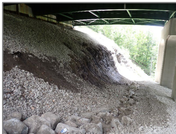
Photo 47 – Erosion channel in front of the Forward Abutment, looking east. Note that new slope protection should mitigate further erosion.
