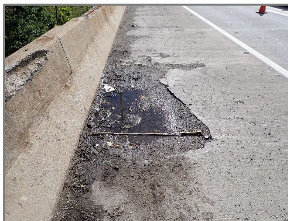
Photo 13 – Large pothole in the right shoulder of the Span 8 wearing surface on the westbound structure at the base of the bridge railing, looking east.
