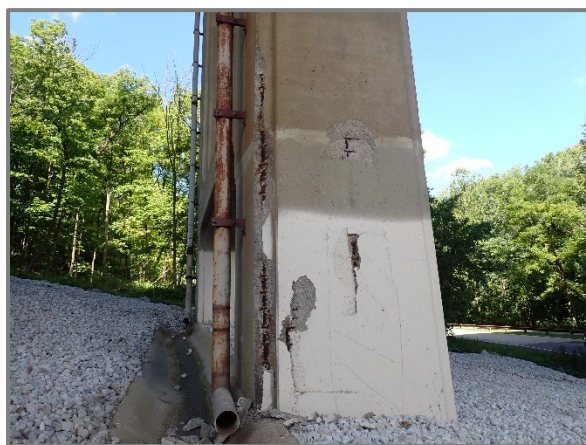
Photo 38 – Numerous spalls with exposed reinforcement on the south column at Pier 2 of the westbound structure, looking northeast.
