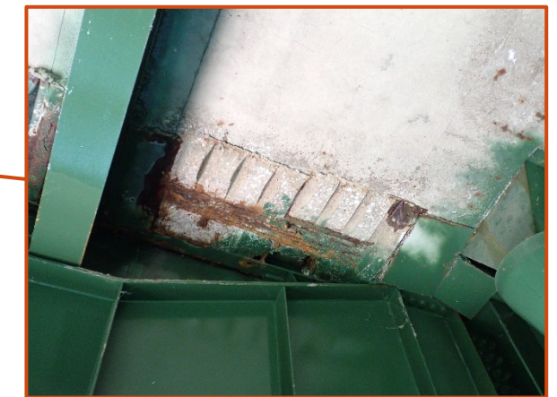
18" long by 8" wide by full depth spall with exposed and corroded reinforcement in the westbound structure deck underside along the Span 4 expansion joint, looking west.
