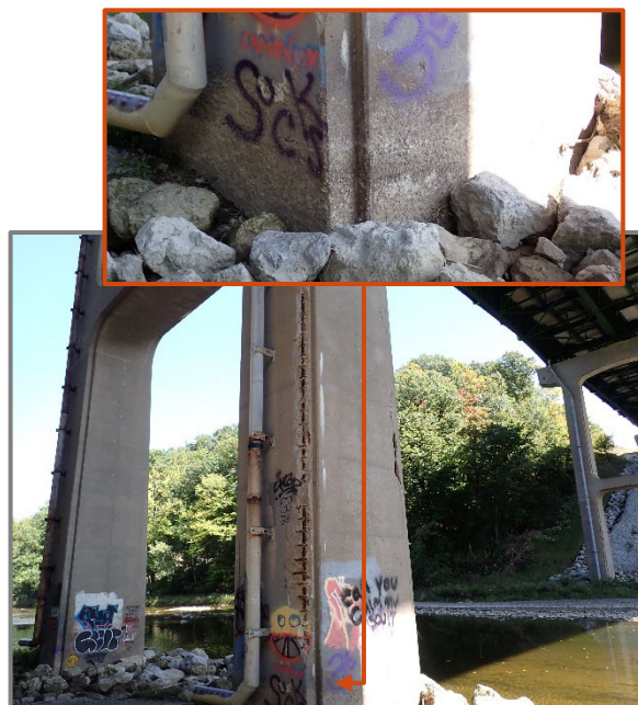
Photo 41 – Corner spalls with exposed reinforcing on south column of Pier 6 of the westbound structure, looking northeast. Note minor scaling to bottom 18" of column.
