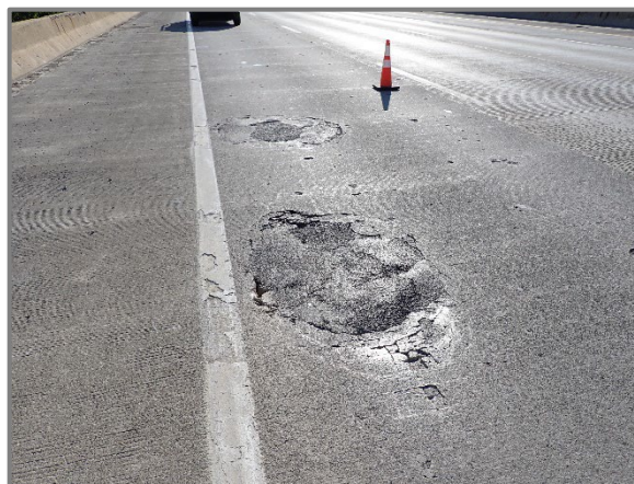
Photo 10 – Typical failing patches in the right lane of the westbound structure wearing surface in Span 5, looking east. Note additional broken up wearing surface material around the perimeter of the patches.
