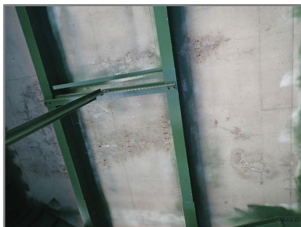
Photo 4 – Several areas of moisture staining and efflorescence in the deck underside between Girders E and F between Floorbeams 43 and 44, looking west. Note these are defects are typically located between failing patches in the wearing surface.
