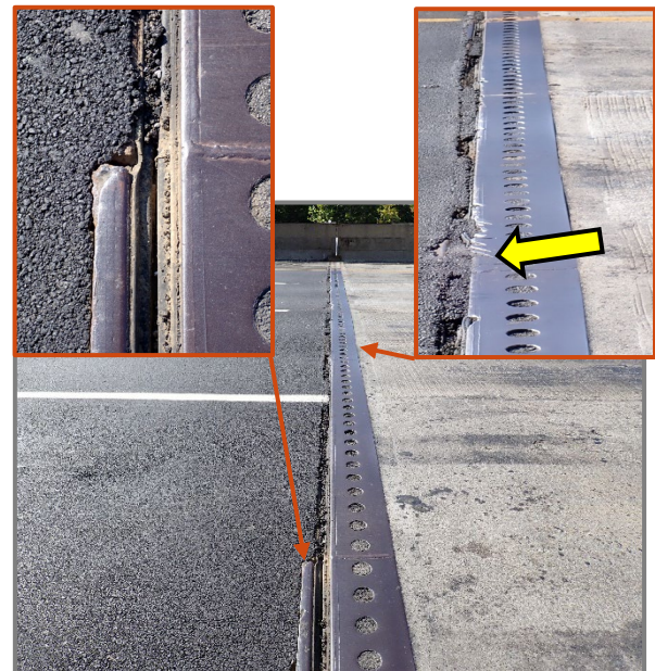
Photo 17 – Westbound Forward Abutment joint with moderate plow damage to the west joint armor and break in the east armor in the right shoulder, looking south. Note east approach has been repaved since the previous inspection and asphalt now covers majority of east joint armor.
