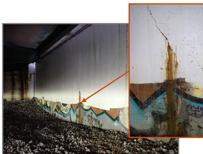
Photo 46 – 1/8" wide vertical/diagonal crack with moderate efflorescence and rust staining in the interior wingwall at the Rear Abutment, looking northwest.
