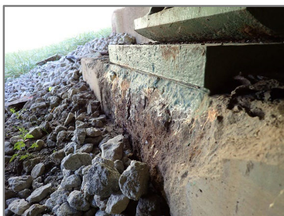
Photo 34 – Spall in the west face of the Girder F seat pedestal at the Forward Abutment undermining the bearing masonry plate up to 3/4" deep, looking north.
