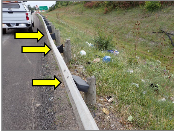
Photo 52 – Damaged timber posts and plastic blockouts on Posts 3 through 6 from the bridge end in the southeast corner approach guardfence, looking east.
