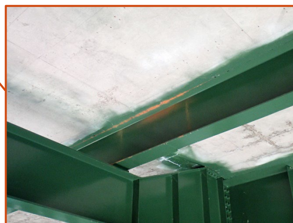
Minor abrasion rust along the top flange of Stringer 9 at Floorbeam 34, looking northwest.
