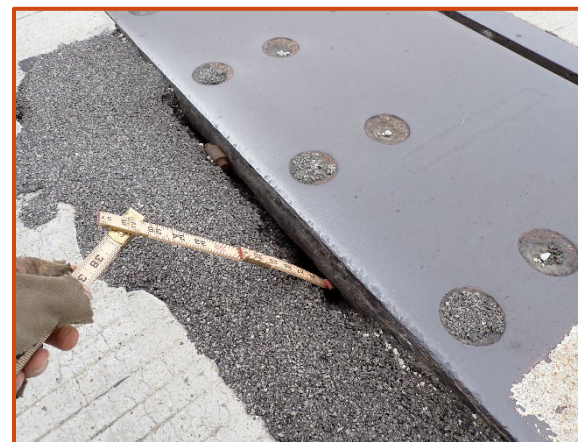
Patching and potholes along west side of Span 6 hinge joint with a 2' wide by 3" long full depth pothole in the right lane of the eastbound structure, looking northeast.
