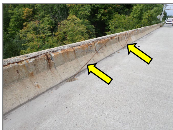
Photo 18 – Typical spalls, up to full width, with exposed, corroded, missing, and debonded reinforcement along the top edges of the exterior bridge railings, looking southwest at the south railing in Span 1 of the eastbound structure. Note the debonded top longitudinal bars hanging down.
