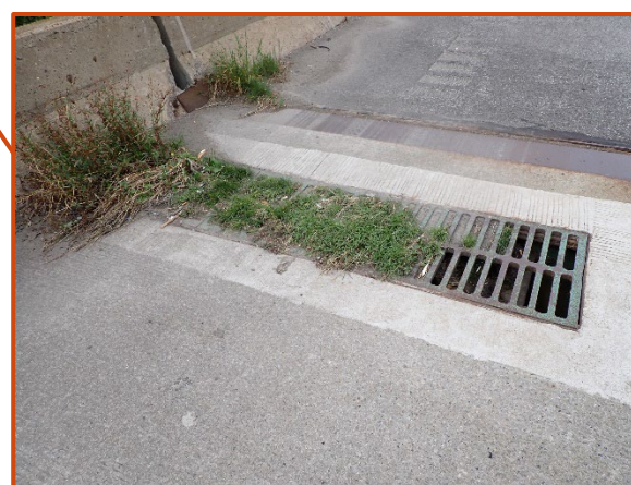
Partially clogged drainage scupper (approximately 85% clogged), looking southwest at the west end of the bridge on the eastbound structure. Note downspout is clear.
