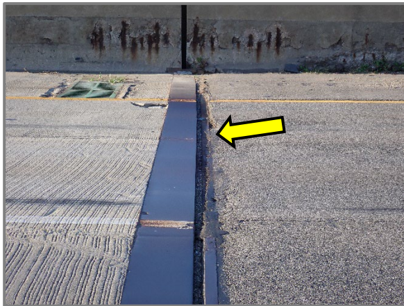
Photo 15 – Joint armor discontinuous and depressed approximately 1/2" at the westbound Rear Abutment joint in the 2 nd lane (from left), looking south.
