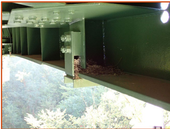
Typical bird nest on top of the girder bottom flange at the retrofit plate, looking southeast.
