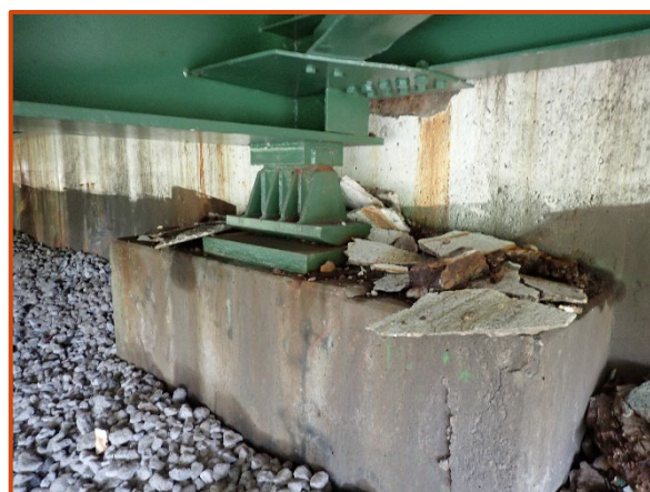
General view of Girder B bearing at the Forward Abutment, looking northeast. Note spalled concrete from backwall behind girder end.
