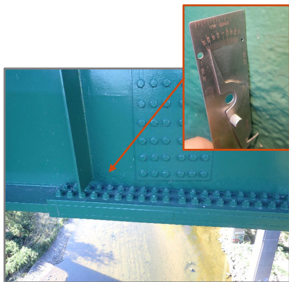
Photo 28 – Cleaned and painted pitting 1/8" deep on the bottom of the north face of the Girder F web along the bolted splice between Floorbeams 54 and 55, looking south.
