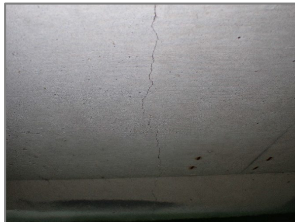
Photo 3 – Typical crack transverse crack, up to 0.020" wide, in the Span 4 underside of deck between Floorbeams 24 and 25 of the eastbound structure, looking north.
