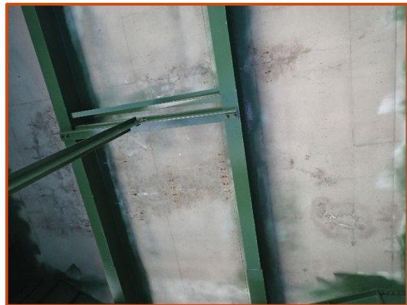
Several areas of moisture staining and efflorescence in the deck underside between Girders E and F between Floorbeams 43 and 44, looking west.
