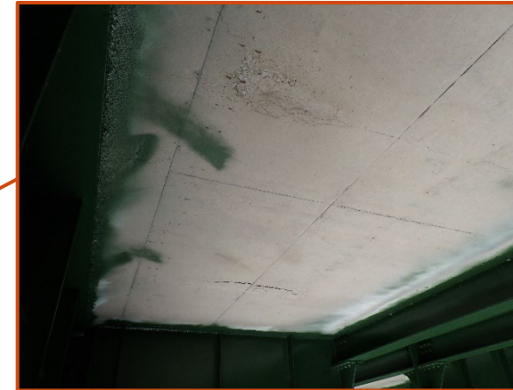
Delaminations in the north deck overhang of the eastbound structure between Floorbeams 64 and 65, looking west.
