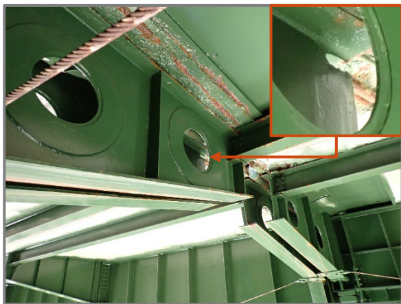
Photo 30 – 3" long by 1" high corrosion hole at the top of the Floorbeam 26 north cantilever on the eastbound structure at its end, looking northwest. Note that Floorbeam 27 is similar.
