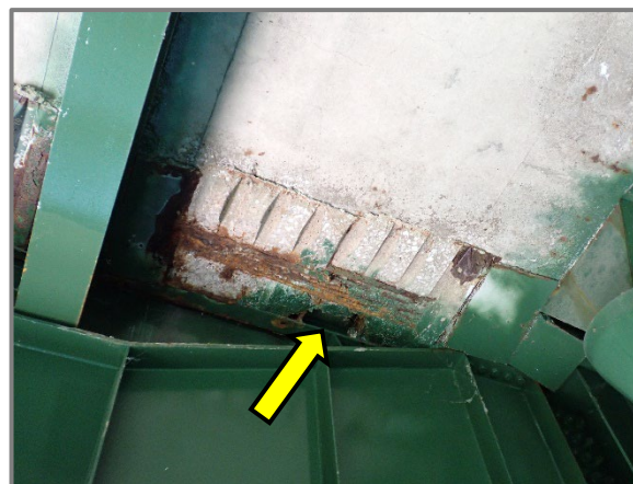
Photo 8 – 18" long by 8" wide by full depth spall with exposed and corroded reinforcement in the westbound structure deck underside along the Span 4 expansion joint, looking west.
