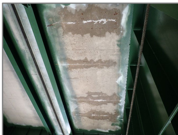
Photo 5 – Typical hairline transverse cracks with light efflorescence and leakage in the deck overhangs, looking west at the south overhang of the westbound structure between Floorbeams 23 and 24.
