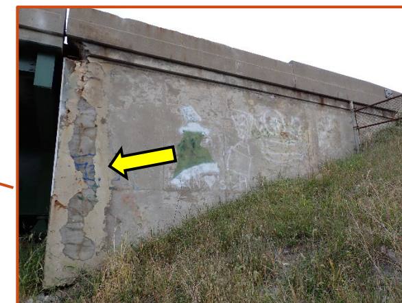
12" wide patch beginning to fail in the south wingwall at the along the Forward Abutment connection, looking north.
