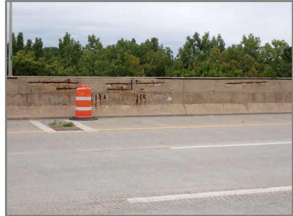
Photo 20 – Widespread spalling of the median barrier on the eastbound structure near Pier 4, looking north.
