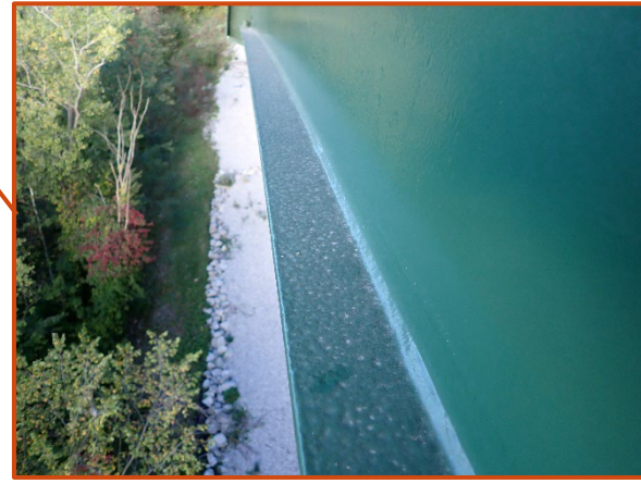
Less than 1/16" deep cleaned and painted pitting on the top face of the Girder A bottom flange on the exterior face between Floorbeams 16 and 18, looking west.
