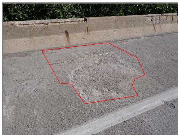
Photo 13 – Delaminated area with moderate abrasion, up to 7'-3" long by 9' wide, in westbound right shoulder, looking north.
