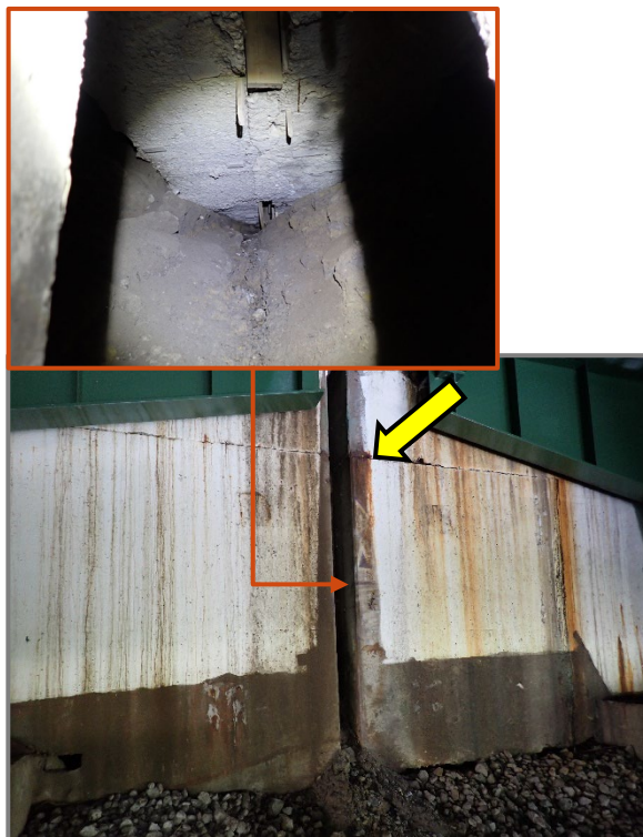
Photo 51 – Embankment fill spilling out from behind the Forward Abutment backwall through the median joint, looking north. Note this embankment fill is located below the reinforced concrete “abutment span” behind this backwall.
