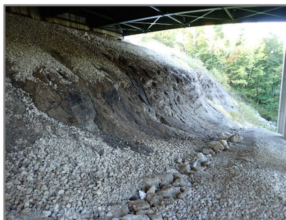
Photo 49 – Erosion channel in front of the Forward Abutment, looking south. Note that new slope protection should mitigate further erosion.
