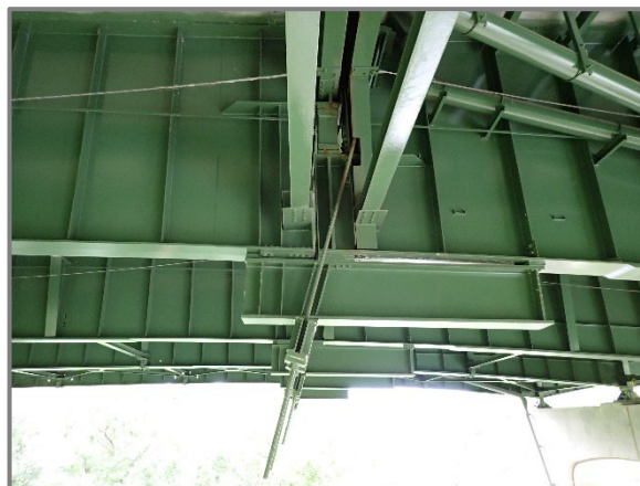
Photo 37 – Typical carrier beam retrofit installed below the seated hinge joints, looking north at Girder C at the Span 6 expansion joint.
