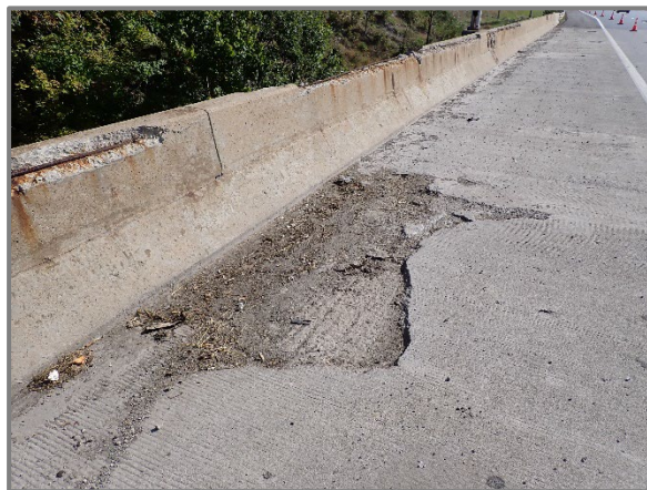
Photo 12 – Large pothole in the right shoulder of the Span 8 wearing surface on the westbound structure at the base of the bridge railing, looking northeast.
