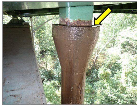
Photo 26 – Downspout at Pier 4 for the eastbound bridge full of water at the time of inspection, looking south.
