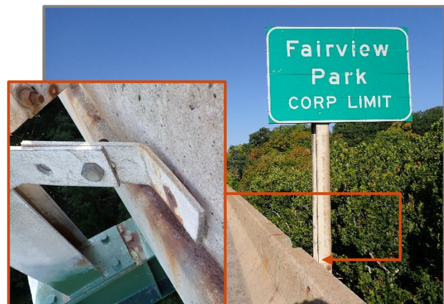
Photo 53 – Broken bolt connecting the "Corporation Limit" to the north rail of the westbound structure in Span 4, looking west. Note sign support still connected to floorbeam top flange.
