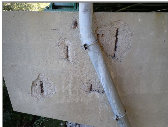
Photo 42 – 72" high by 60" wide area with that is delaminated and spalled up to 2" deep with exposed and corroded reinforcement behind the downspout on the west face of the Pier 7 cap for the westbound structure, looking east.
