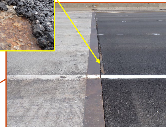
Up to 1" vertical misalignment at the eastbound Forward Abutment joint in the right two lanes, looking north. Note the asphalt on the east side of the joint has been replaced since the previous inspection.
