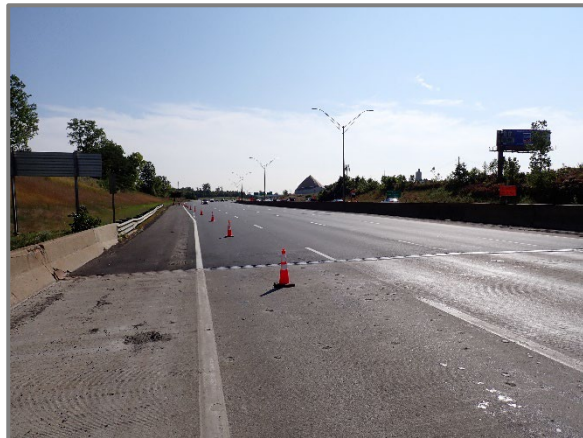
Photo 50 – Forward approach roadway resurfaced since the previous inspection, looking east.
