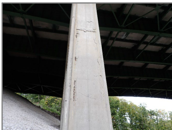
Photo 40 – Numerous spalls with exposed reinforcement and delaminations on the south column at Pier 1 of the eastbound structure, looking north.
