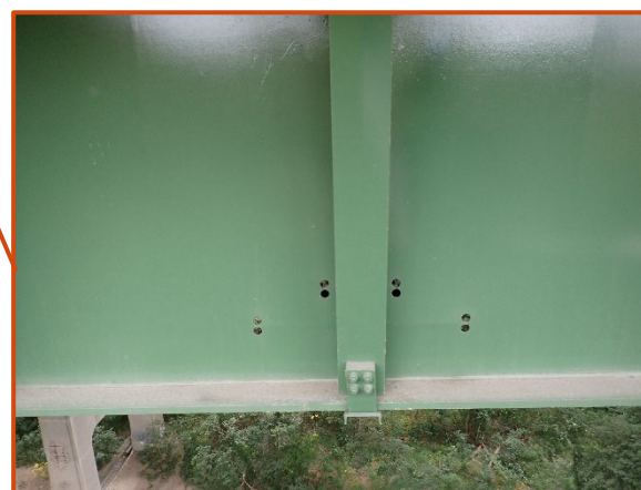
General view of dogbone retrofits in Girder A at Floorbeam 37, looking north.
