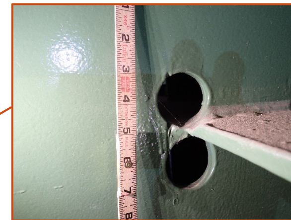
Typical dogbone retrofit overcut in the girder web, looking north at Girder B at Floorbeam 6.
