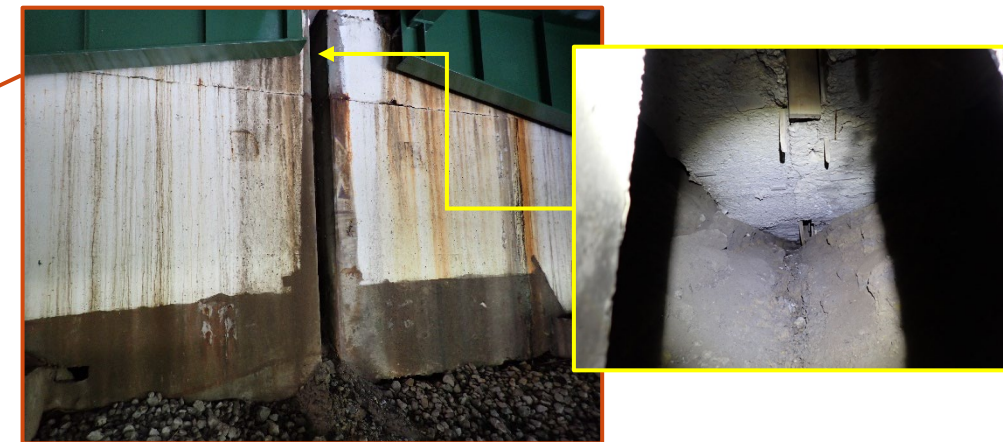
Embankment fill spilling out from behind the Forward Abutment backwall through the median joint, looking north. Note the 8' tall by 15' wide by 30' deep void that has resulted below the approach slabs with an active runoff erosion channel.
