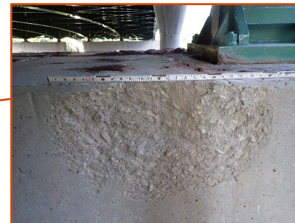
Top corner spall with exposed reinforcement in the east face of the Pier 7 cap on the westbound structure, looking west.
