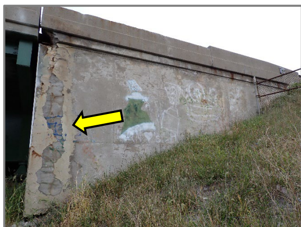
Photo 45 – 12" wide patch beginning to fail in the south wingwall at the along the Forward Abutment connection, looking north.
