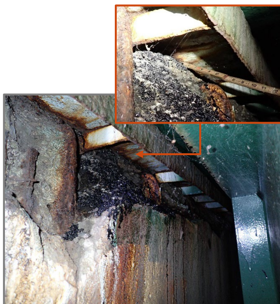
Photo 43 – 12" high by 10" deep by 8.5' wide spall with exposed reinforcement in the top of the Forward Abutment backwall behind Girder C that is undermining the joint armor support up to 10", looking southeast. Note this area is under the left shoulder of the eastbound bridge.
