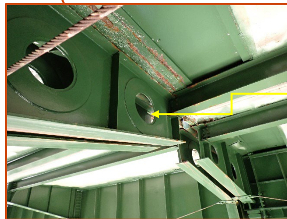
3" long by 1" high corrosion hole at the top of the Floorbeam 26 north cantilever on the eastbound structure at its end, looking northwest.
