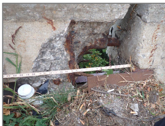
Photo 19 – 24" long by 24" high by full depth spall in the south bridge railing on the east side of the Span 6 joint on the eastbound structure, looking south. Note that spalls of this nature are typically present at the hinge joints.
