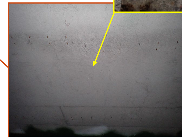
Typical 0.012" to 0.014" wide map cracking at 6" to 12" spacing in the underside of deck, looking north.
