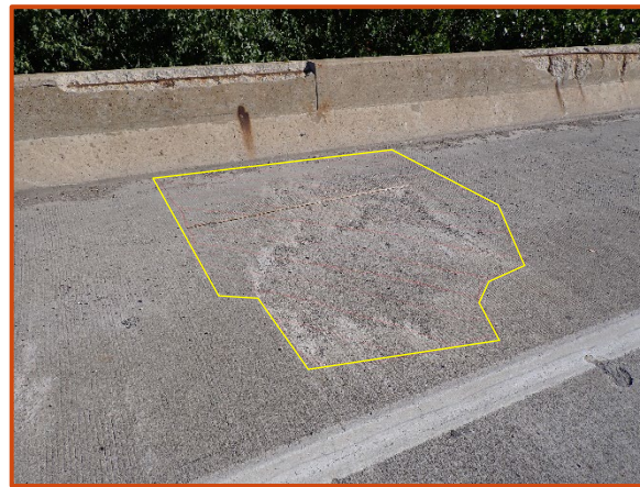
Delaminated area with moderate abrasion, up to 7'-3" long by 9' wide, in westbound right shoulder, looking north.
