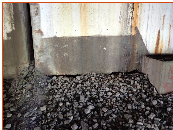
Forward Abutment backwall for the eastbound structure undermined up to 5" high by 13" deep over a 7' length at the north end, looking east.
