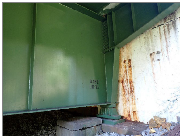
Photo 36 – New stamp denoting the recently applied OZEU protective coating system, looking southwest at Girder F at the Rear Abutment.
