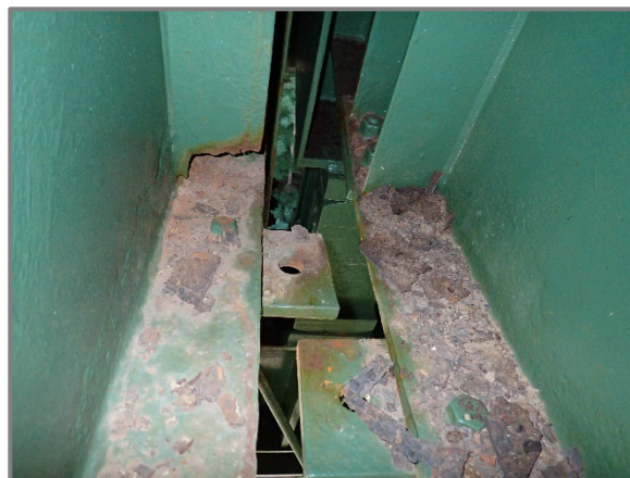
Photo 32– South cantilever of Floorbeam 26 on the westbound structure with 100% section loss at the base of a transverse stiffener near the base, looking north.
