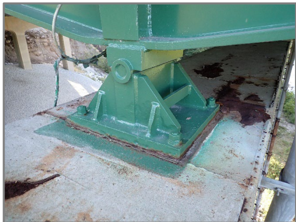
Photo 35 – Up to 1/4" deep cleaned and painted pitting on the bearing assembly and masonry plate for Girder F at Pier 7, looking south.
