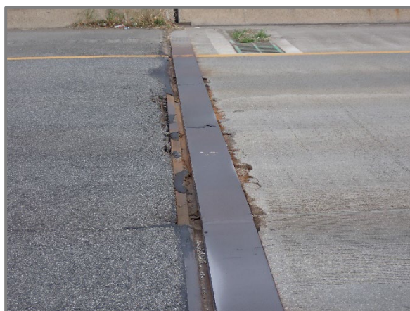
Photo 14 – 1/2" vertical misalignment at the Rear Abutment joint for the eastbound structure, looking north. Note the adjacent spalling to the joint header in the 2 nd lane (from left).
