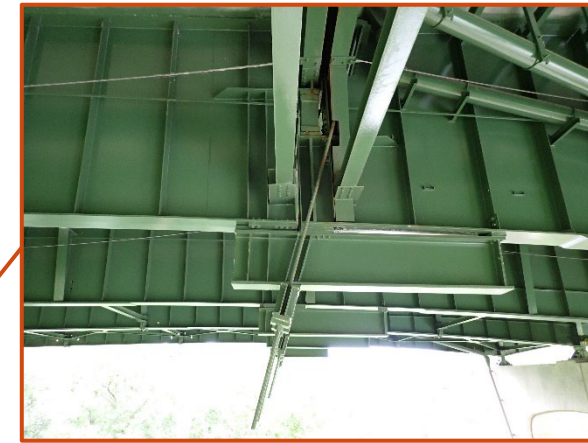
Typical carrier beam retrofit installed below the seated hinge joints, looking north at Girder C at the Span 6 expansion joint.
