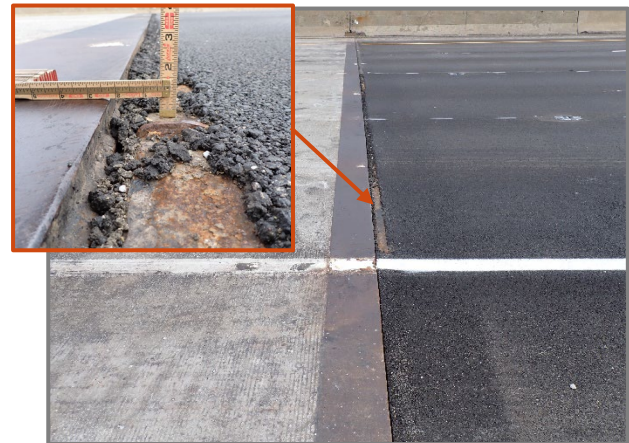
Photo 16 – Up to 1" vertical misalignment at the eastbound Forward Abutment joint in the right two lanes, looking north. Note the asphalt on the east side of the joint has been replaced since the previous inspection.
