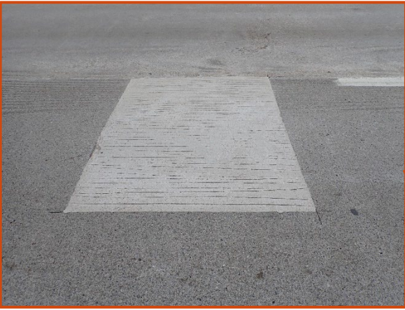
5' long by 6' wide patch in the right lane of the wearing surface in Span 8 of the eastbound structure, looking north.
