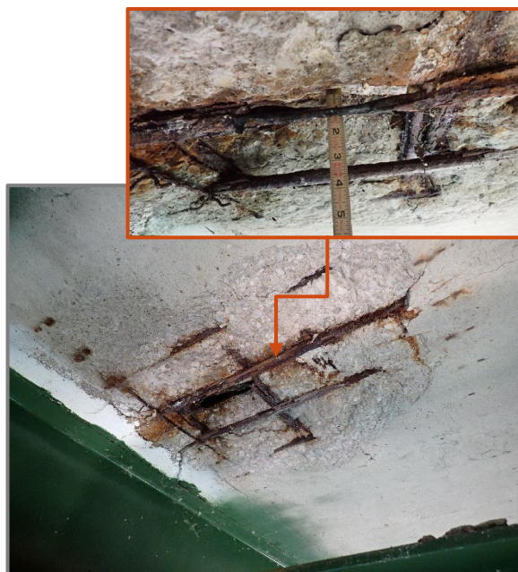
Photo 6 – 36" long by 42" wide by up to 5" deep spall with debonded and corroded reinforcement (up to 90%) along the south side of Stringer 11 at Floorbeam 42 on the westbound structure, looking northeast.
