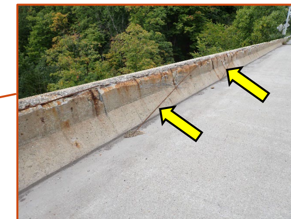
Typical spalls, up to full width, with exposed, corroded, missing, and debonded reinforcement along the top edges of the exterior bridge railings, looking southwest at the south railing in Span 1 of the eastbound structure. Note the debonded top longitudinal bars hanging down.
