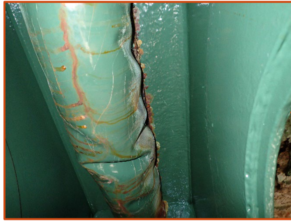
Floorbeam 26 south cantilever on the westbound structure with cleaned and painted pitting 1/8" deep for the full width of the east top flange, looking south.
