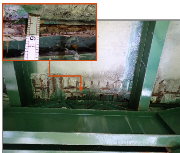
Photo 7 – 7' wide by up to 15" long by full depth spall with two layers of fully exposed and corroded reinforcement at the end of the eastbound structure deck along the Span 6 expansion joint armor, looking east. Note up to 20% section loss to the exposed reinforcement.
