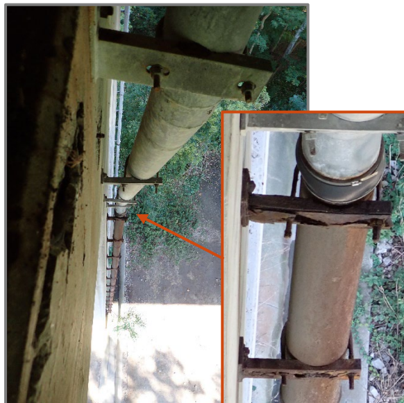
Photo 23 – Downspout on Pier 3 of westbound structure with moderate surface corrosion to downspout pipe and corrosion holes in downspout supports due to leakage from joint, looking north.
