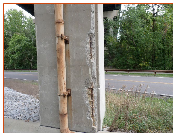
Southwest corner spall with exposed and corroded reinforcement near the base of the south column on Pier 2 of the eastbound structure, looking east.
