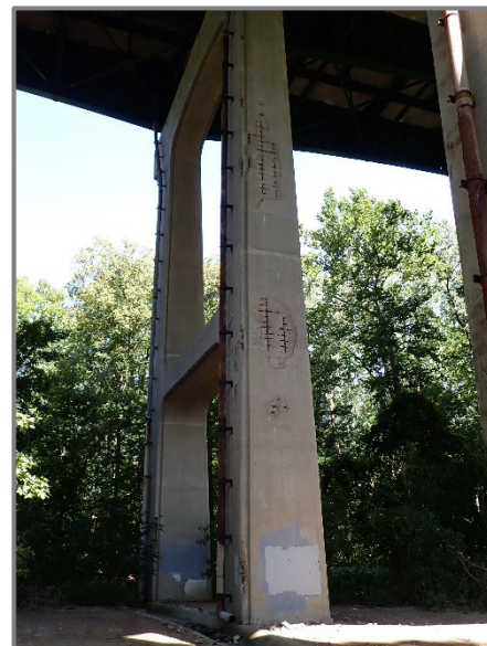
Photo 38 – Numerous delaminations and spalls with exposed reinforcement throughout the north column at Pier 3 of the eastbound structure, looking southwest.
