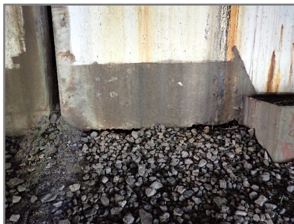
Photo 44 – Forward Abutment backwall for the eastbound structure undermined up to 5" high by 13" deep over a 7' length at the north end, looking east.
