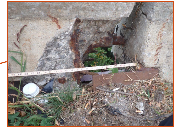
24" long by 24" high by full depth spall in the south bridge railing on the east side of the Span 6 joint on the eastbound structure, looking south. Note that spalls of this nature are typically present at the hinge joints.
