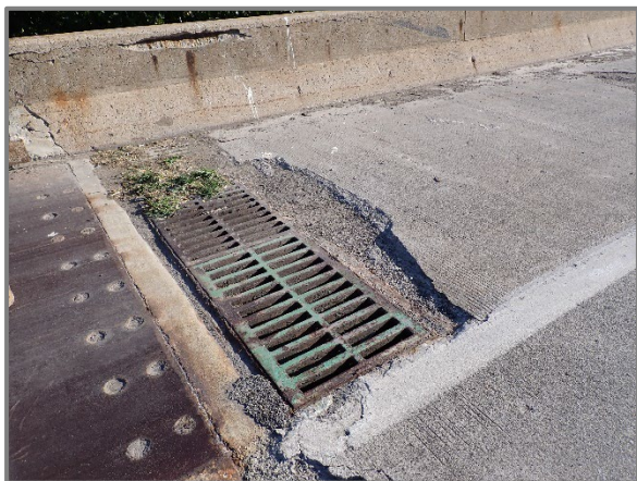
Photo 11 – Typical potholes along the drainage scuppers, looking northeast at a drainage scupper in the westbound right shoulder in Span 4.
