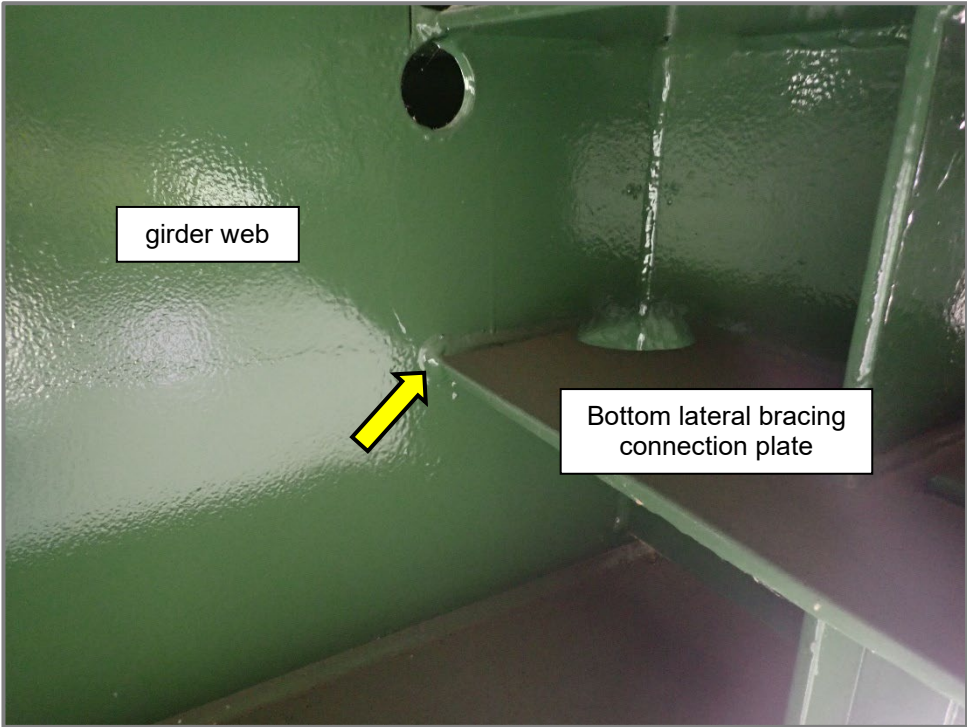
Photo 2 – Base metal at lateral bracing connection plate to girder web welds (Category E). Girder F at Floorbeam 37 shown, looking south.
