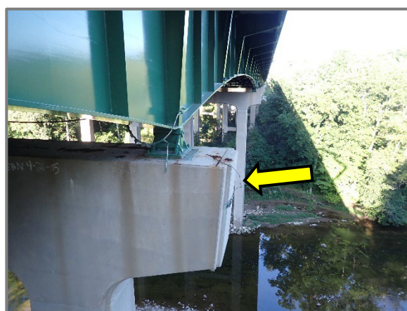
Photo 56 – Typical broken grounding cable at the pier caps, looking west at Pier 7 adjacent to Girder F.
