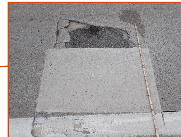
3' long by 1.5' by 3" deep pothole/spall (partially filled with asphalt) in the right lane of the wearing surface in Span 8 of the eastbound structure, looking north.
