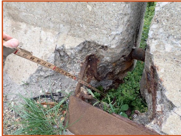
Deck edge and railing spalls with exposed and corroded reinforcement along the Span 4 expansion joint at the south edge of the eastbound structure, looking south.
