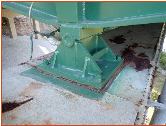
Up to 1/4" deep cleaned and painted pitting on the bearing assembly and masonry plate for Girder F at Pier 7, looking south.
