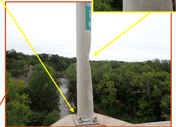
Light post GR1-2-6 at Pier 7 on the eastbound structure with indentation on west face and leaning to the east due to impact. Note east half of base is crimped and the base plate is bent up 1/2".
