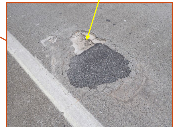
Up to 3 1/2" deep partially patched spall/pothole in the right lane of the Span 4 wearing surface on the eastbound structure, looking northwest.
