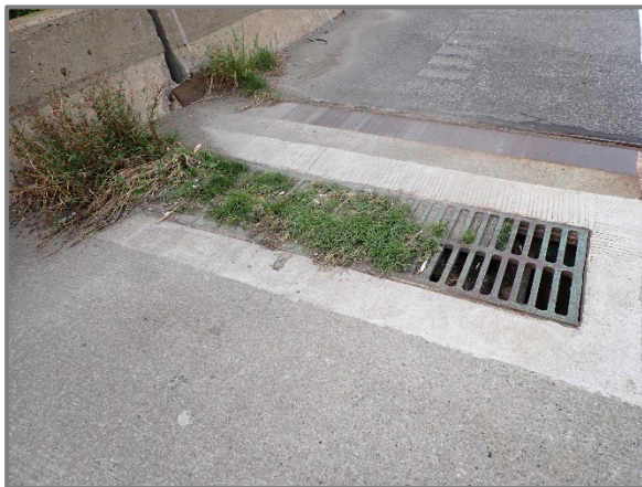
Photo 21 – Partially clogged drainage scupper (approximately 85% clogged), looking southwest at the west end of the bridge on the eastbound structure. Note downspout is clear.
