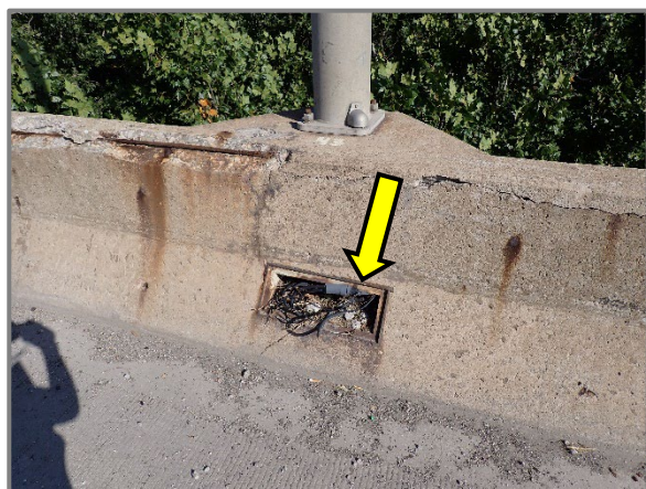
Photo 55 – Typical missing electrical panel access hatch below the light poles, looking north at north railing in Span 6. Note exposed wiring, dirt, granular debris, and vegetation growth inside the panel.
