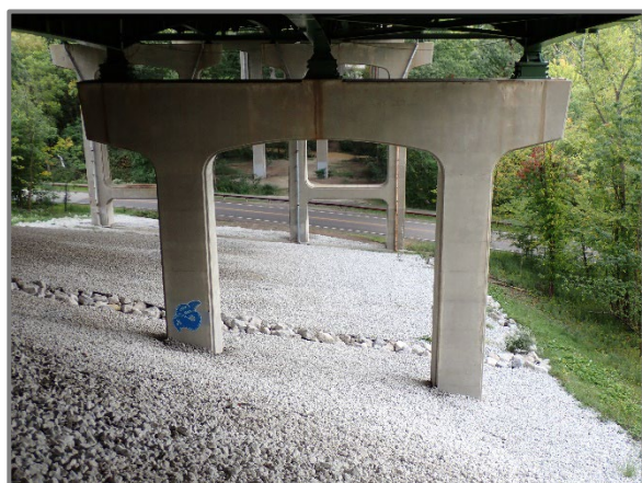
Photo 47 – View of slope protection on west slope from the Rear Abutment, looking east.
