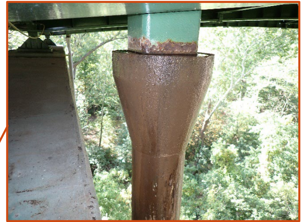
Downspout at Pier 4 for the eastbound bridge full of water at the time of inspection, looking south.
