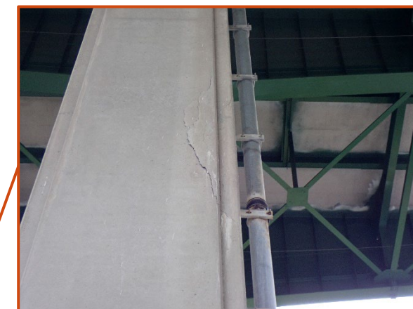
10' high northwest corner delamination on the north face of the south column on Pier 2 of the eastbound structure, looking south.
