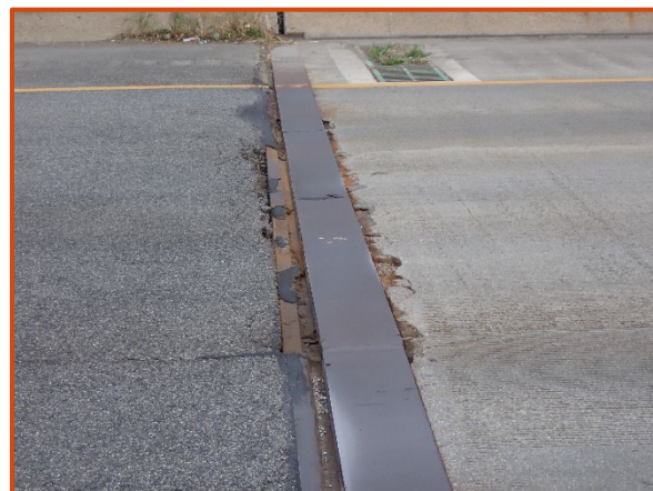
1/2" vertical misalignment at the Rear Abutment joint for the eastbound structure, looking north. Note the adjacent spalling to the joint header in the 2nd lane (from left).
