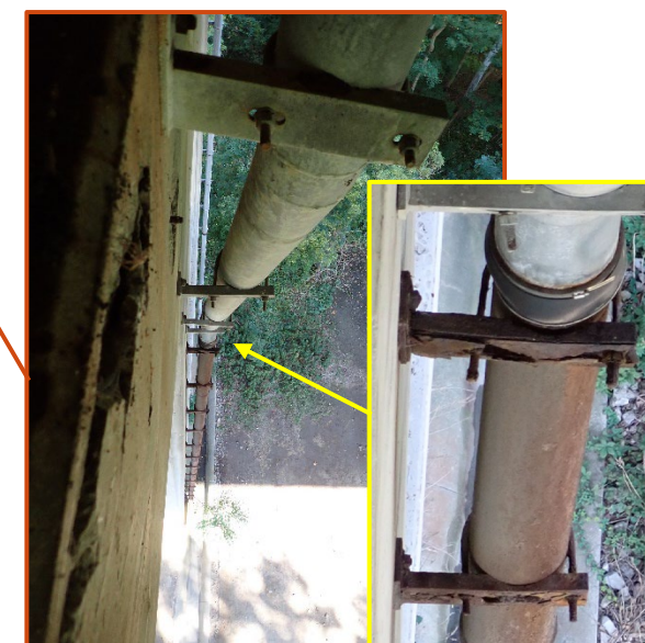
Downspout on Pier 3 of westbound structure with moderate surface corrosion to downspout pipe and corrosion holes in downspout supports due to leakage from joint, looking north.
