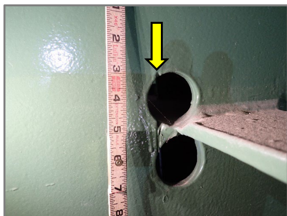
Photo 27 – Typical dogbone retrofit overcut in the girder web, looking north at Girder B at Floorbeam 6.
