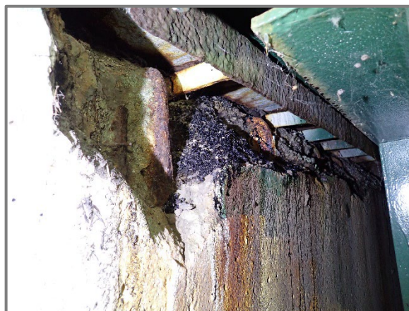
Photo 39 – Spall at the top of the Forward Abutment backwall behind Girder C undermining the joint armor above, looking northeast.
